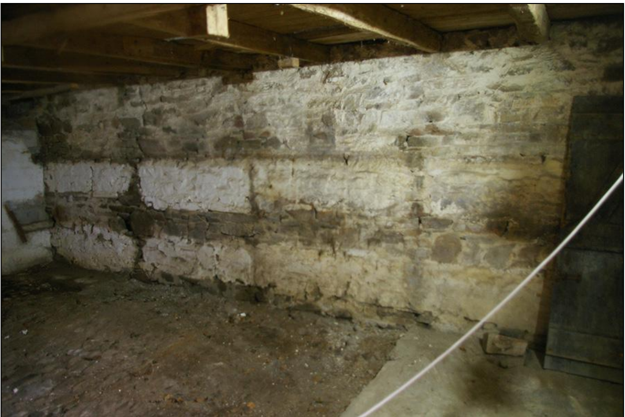
THE SOUTH WALL OF BUILDING 1, WITHIN THE WEST COMPARTMENT, AS VIEWED FROM THE NORTH-WEST CORNER.
