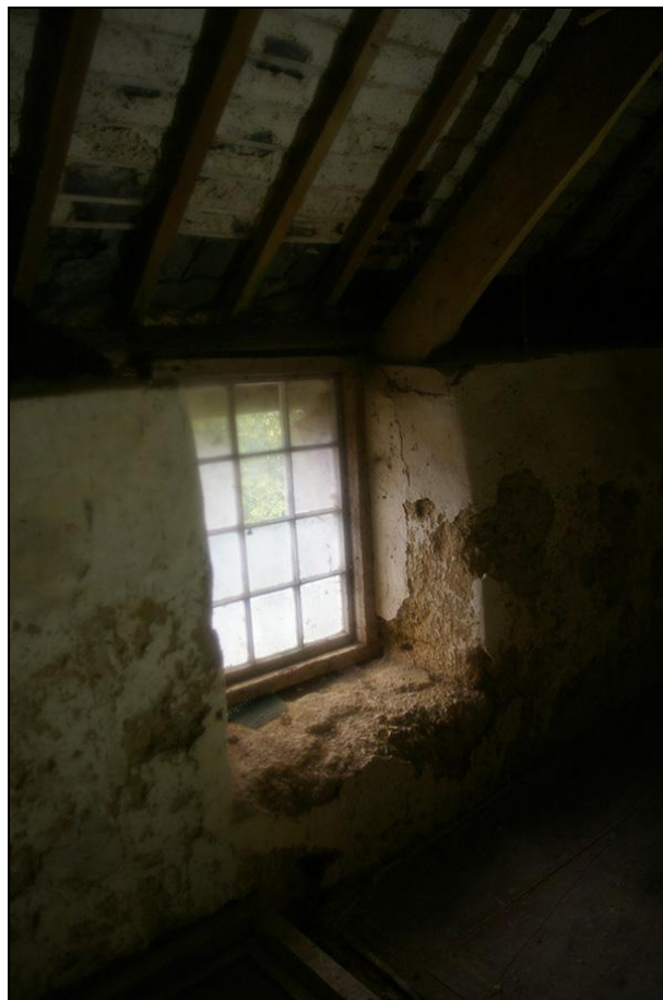
THE FORCED WINDOW IN THE EAST END OF THE LOFT IN BUILDING 1, WITH INSET RECYCLED SASH WINDOW; FROM THE SOUTH-WEST.
