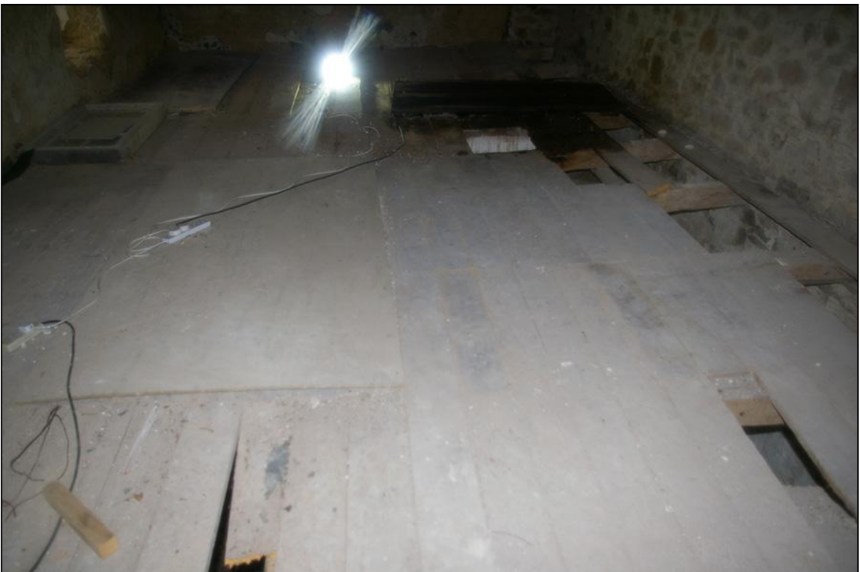
THE LOFT FLOOR, WHICH HAS FAILED AND IS VERY ROTTEN DUE TO ISSUES WITH THE ROOF IN THE PAST; FROM THE WEST.
