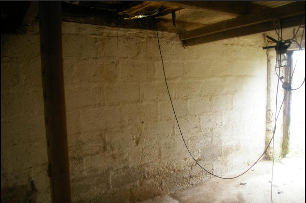
THE CONCRETE PARTITION WALL WHICH SEPARATES THE EASTERN COMPARTMENT FROM THE REST OF THE GROUND FLOOR OF BUILDING 1; FROM THE SOUTH-EAST.
