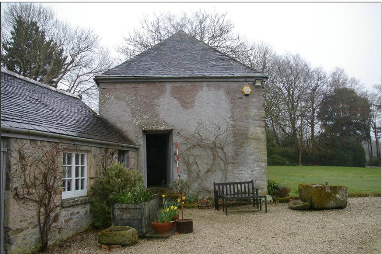
THE WEST ELEVATION OF BUILDING 1, SHOWING THE ADJOINING OUTBUILDING RANGE AND HOW THE GROUND LEVELS HAVE BEEN LOWERED ON THIS SOUTH SIDE, WITH 2M SCALE; FROM THE WEST.
