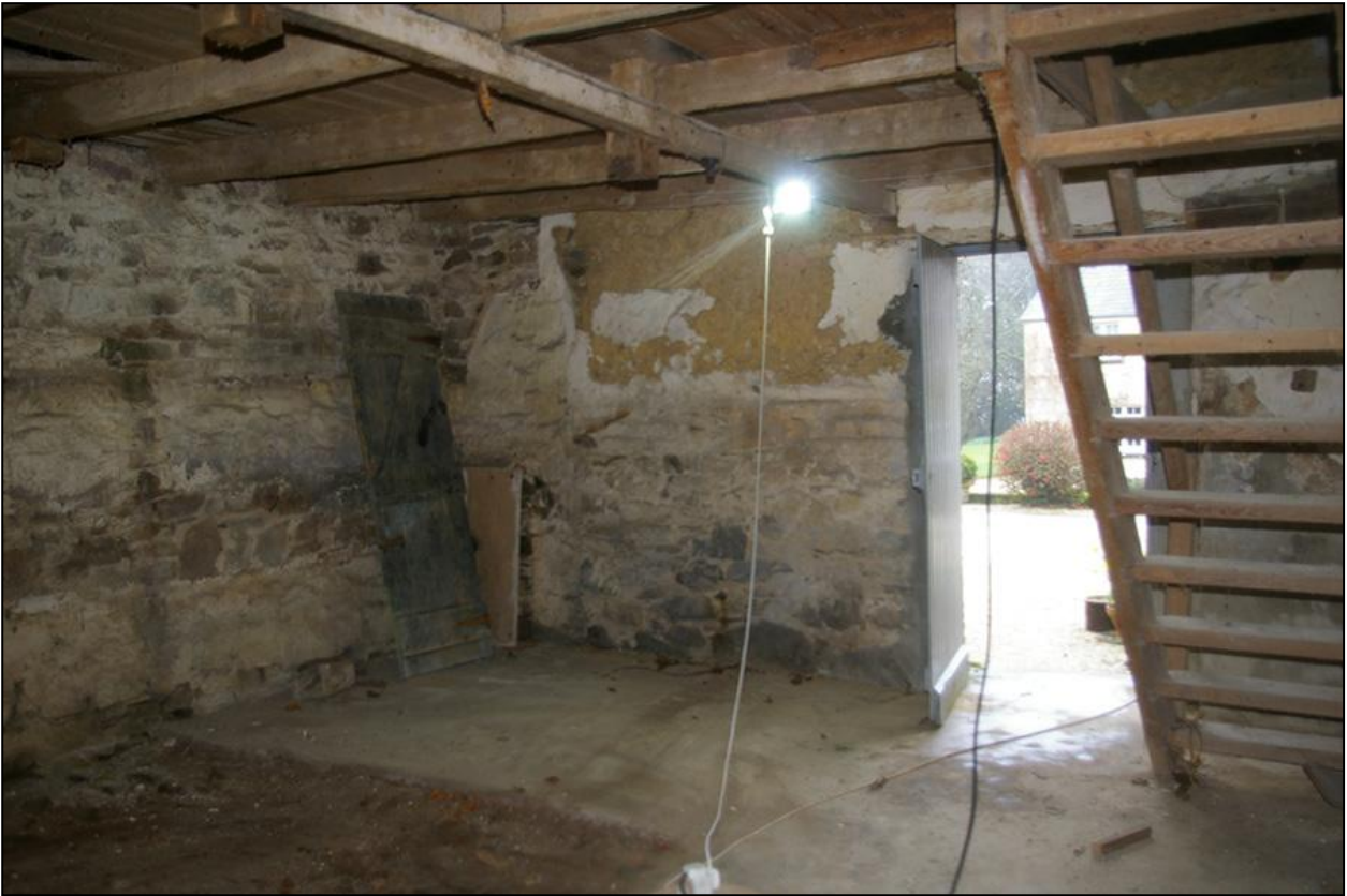
THE WEST ELEVATION OF BUILDING 1 AND WEST END OF THE WEST COMPARTMENT; FROM THE EAST, NORTH-EAST.
