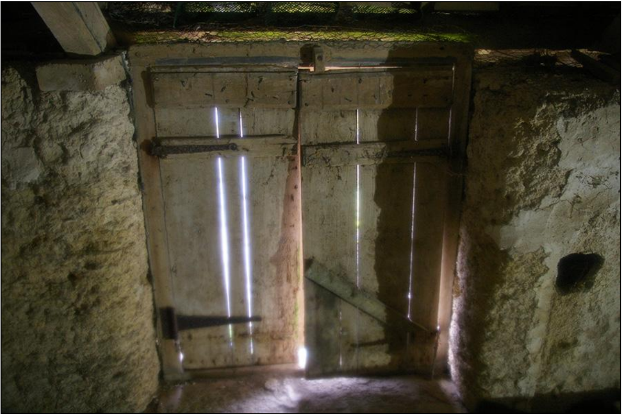
THE LOADING DOOR IN THE NORTH WALL AT LOFT HEIGHT, IN BUILDING 1; FROM THE SOUTH.
