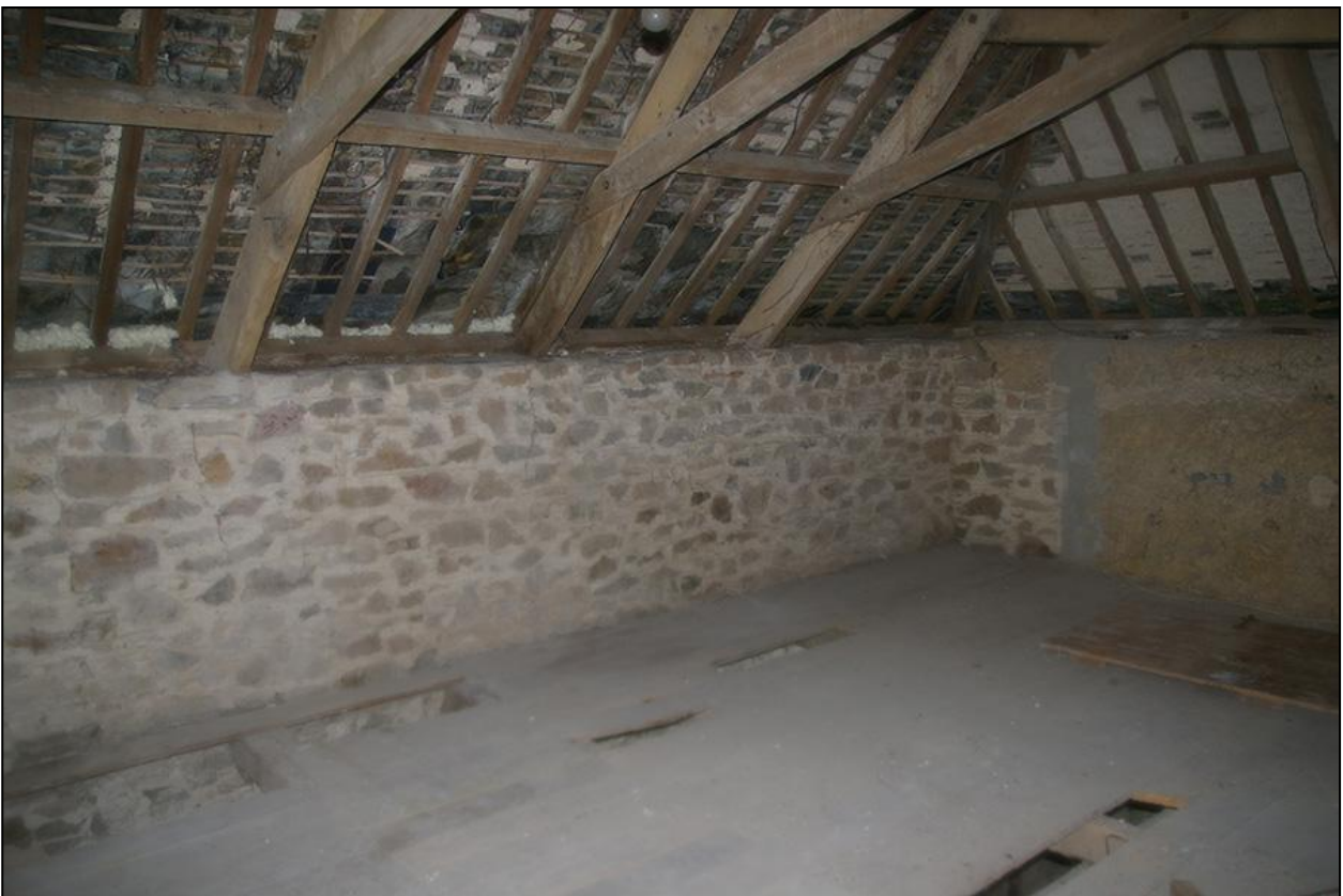
THE SOUTH WALL AND SOUTH-WEST CORNER OF BUILDING 1; FROM THE NORTH EAST.
