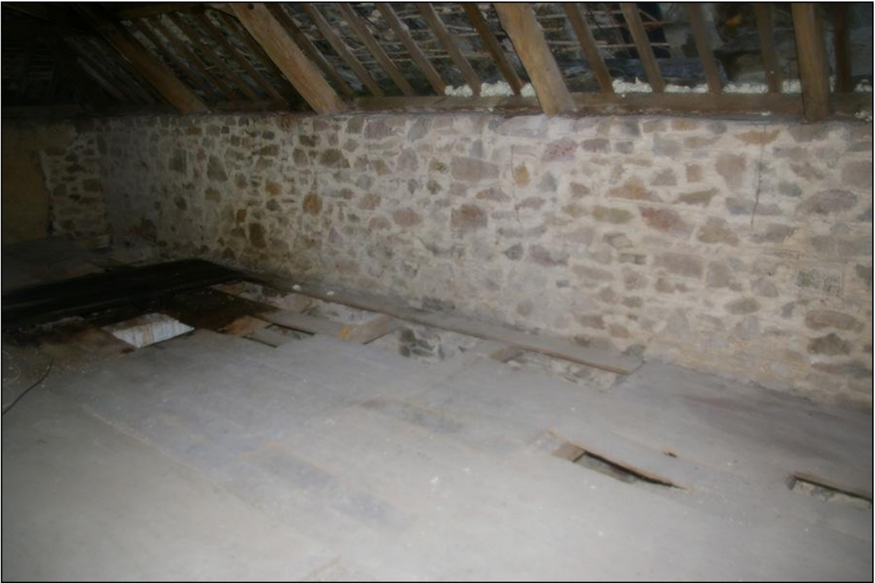
THE SOUTH WALL AND SOUTH-EAST CORNER FROM THE NORTH-WEST CORNER OF THE LOFT.
