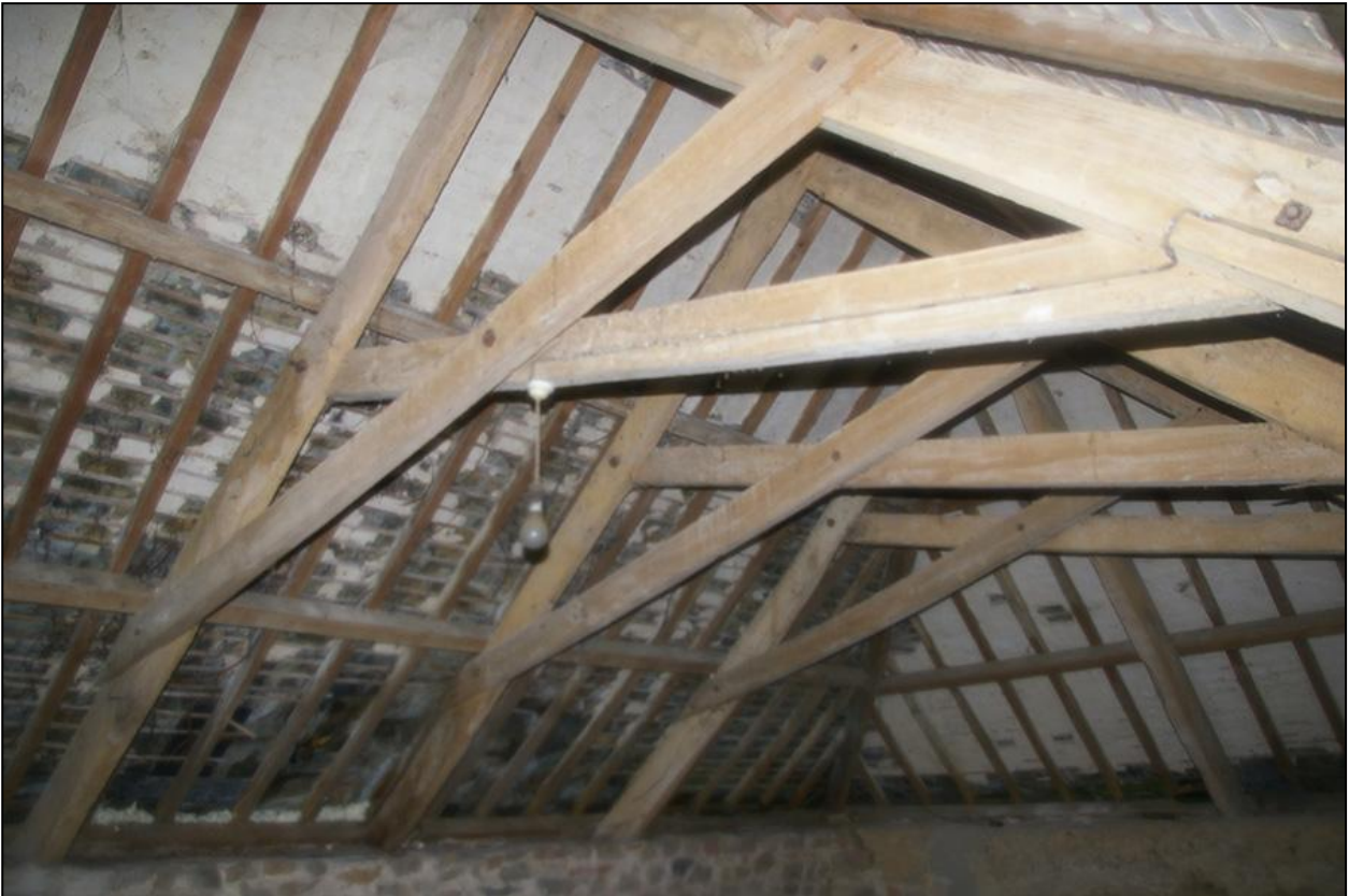
THE ROOF OF BUILDING 1, SHOWING THE TORCHING UNDERNEATH THE SLATES; FROM THE NORTH, NORTH-EAST.
