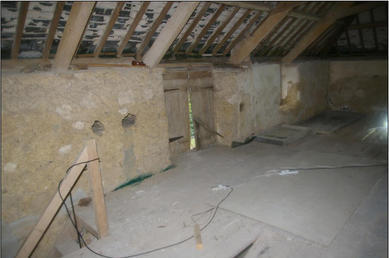
THE NORTH WALL, WITH DOVE HOLES, LOADING DOOR AND FORCED WINDOW TO THE EAST END, SHOWING THE RAISE IN THE COLOUR AND TEXTURE DIFFERENCE IN THE COB FOR THE TOP C.0.4M; FROM THE SOUTH-WEST.
