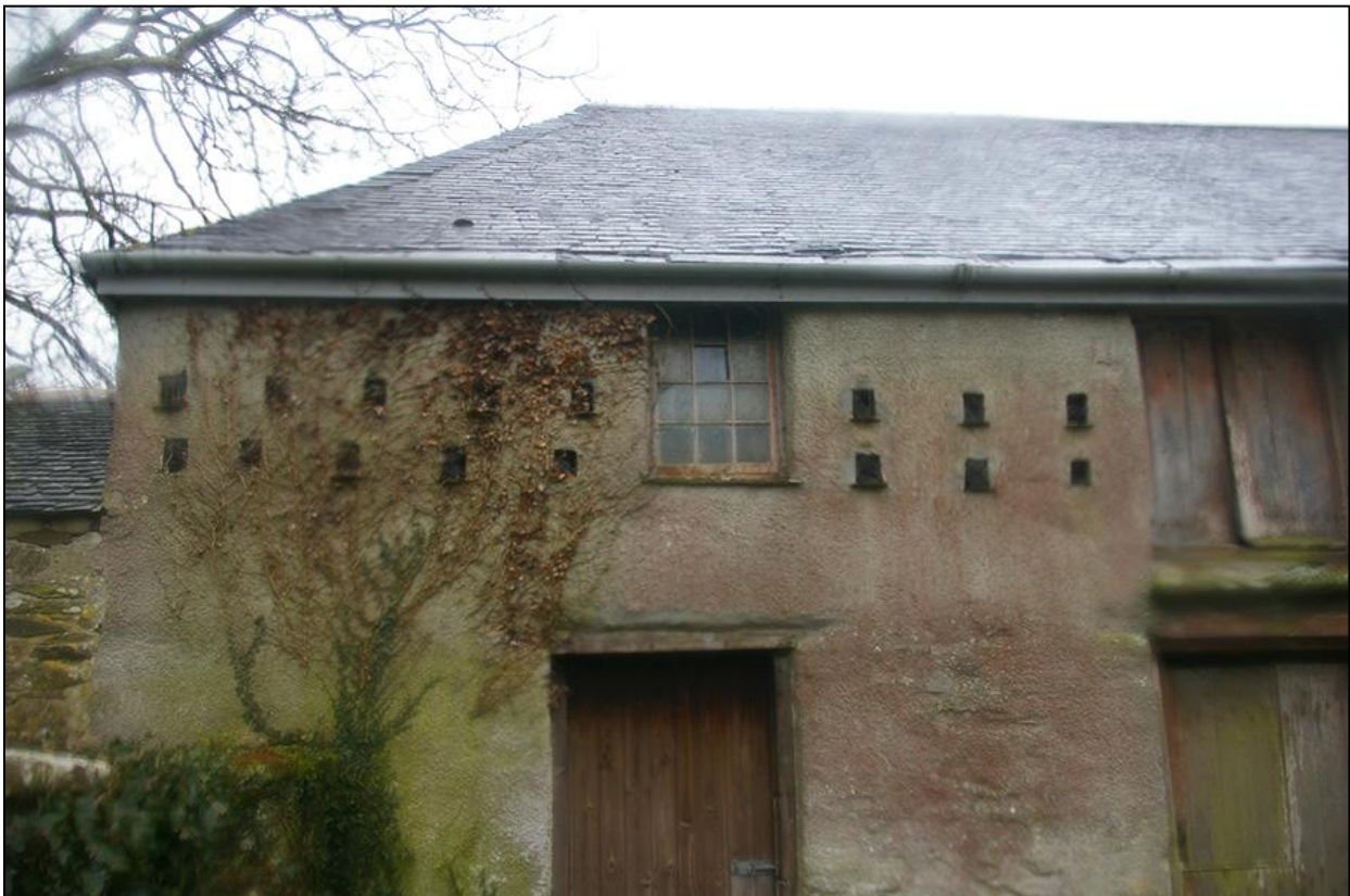
THE ROWS OF DOVE HOLES IN THE NORTH ELEVATION OF BUILDING 1, THOSE TO THE EAST; FROM THE NORTH.
