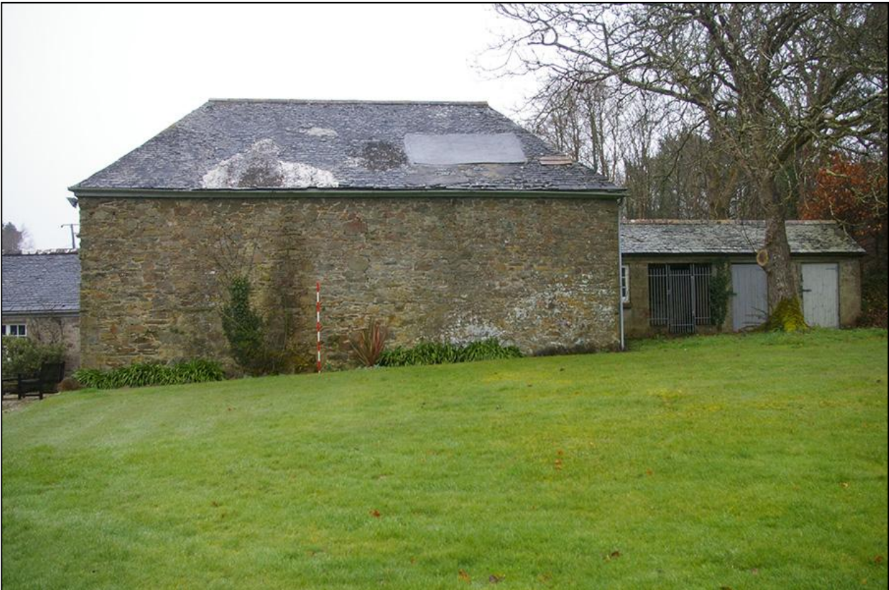
THE SOUTH ELEVATION OF THE BARN, BUILT OF STONE RUBBLE, WITH 2M SCALE; FROM THE SOUTH.
