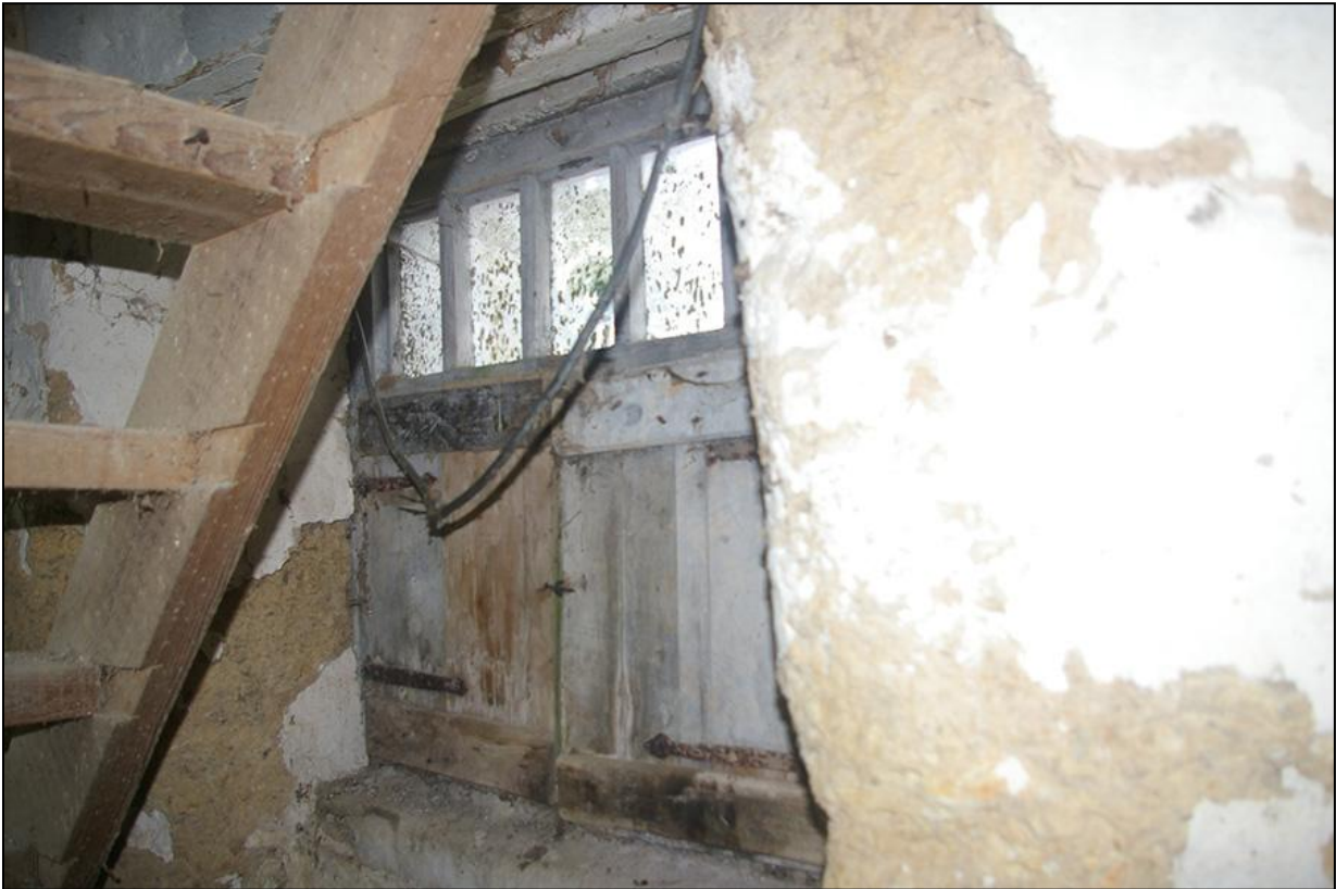
THE WINDOW, SET WITHIN THE BLOCKED DOORWAY; FROM THE SOUTH-EAST AND SOUTH.
