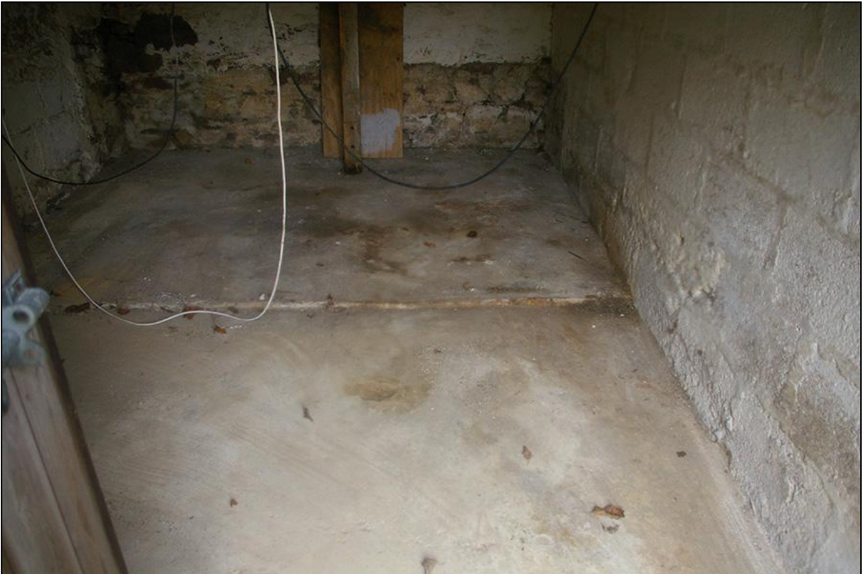
THE CONCRETE FLOOR OF THE EASTERN COMPARTMENT IN BUILDING 1; FROM THE NORTH, NORTH-WEST.
