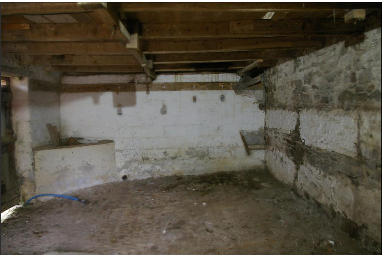
THE WEST LARGER COMPARTMENT WITHIN BUILDING 1, LOOKING TOWARDS THE CONCRETE PARTITION WALL; FROM THE WEST.
