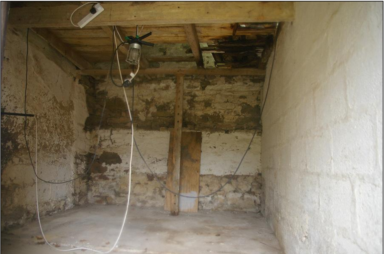
THE NARROW EASTERN COMPARTMENT ON THE GROUND FLOOR OF BUILDING 1; FROM THE NORTH.
