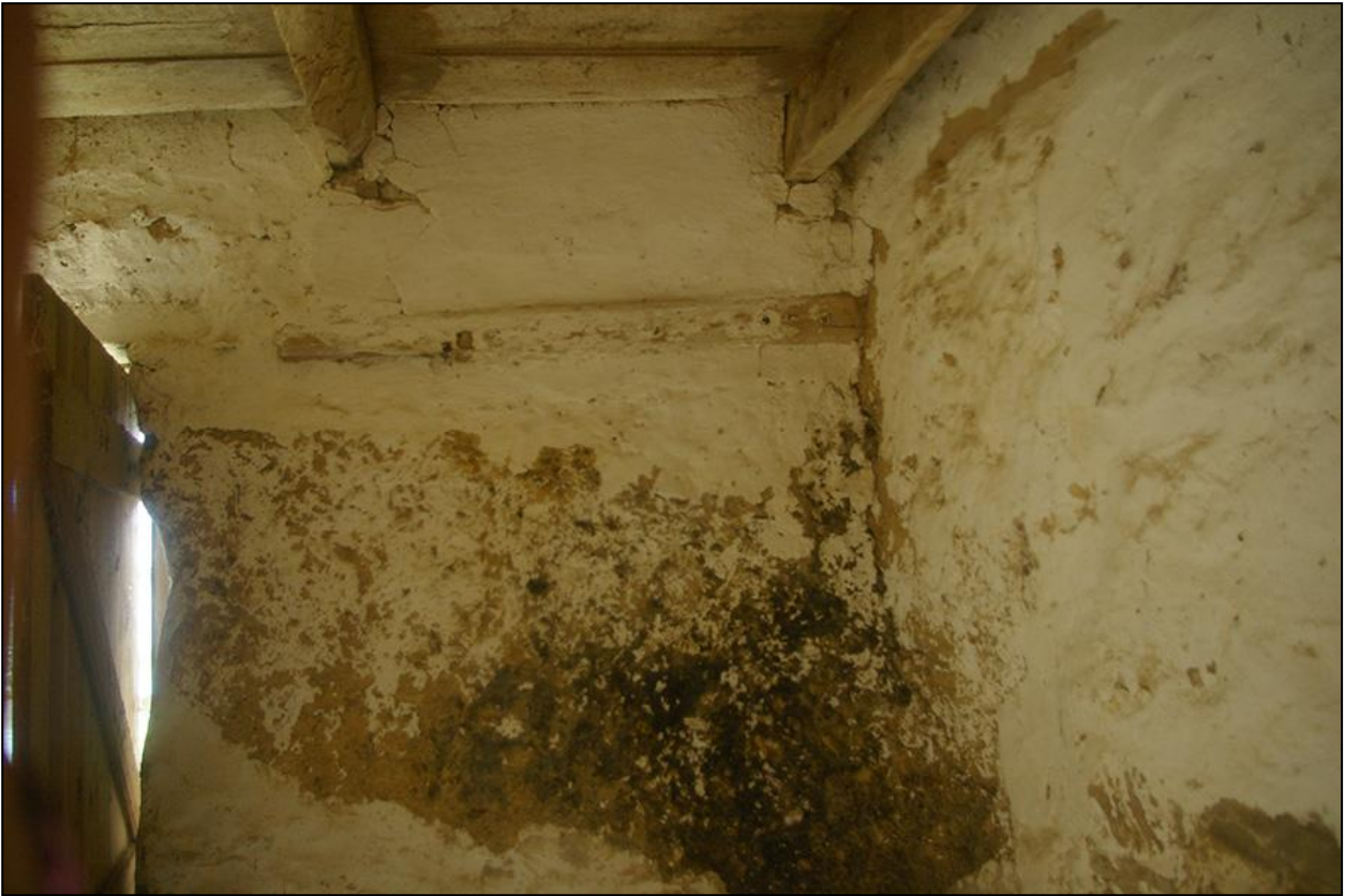
TIMBER TIE, OR FORMER LINTEL IN THE NORTH-EAST CORNER OF BUILDING 1, PART OF A FORMER HAYRACK?
