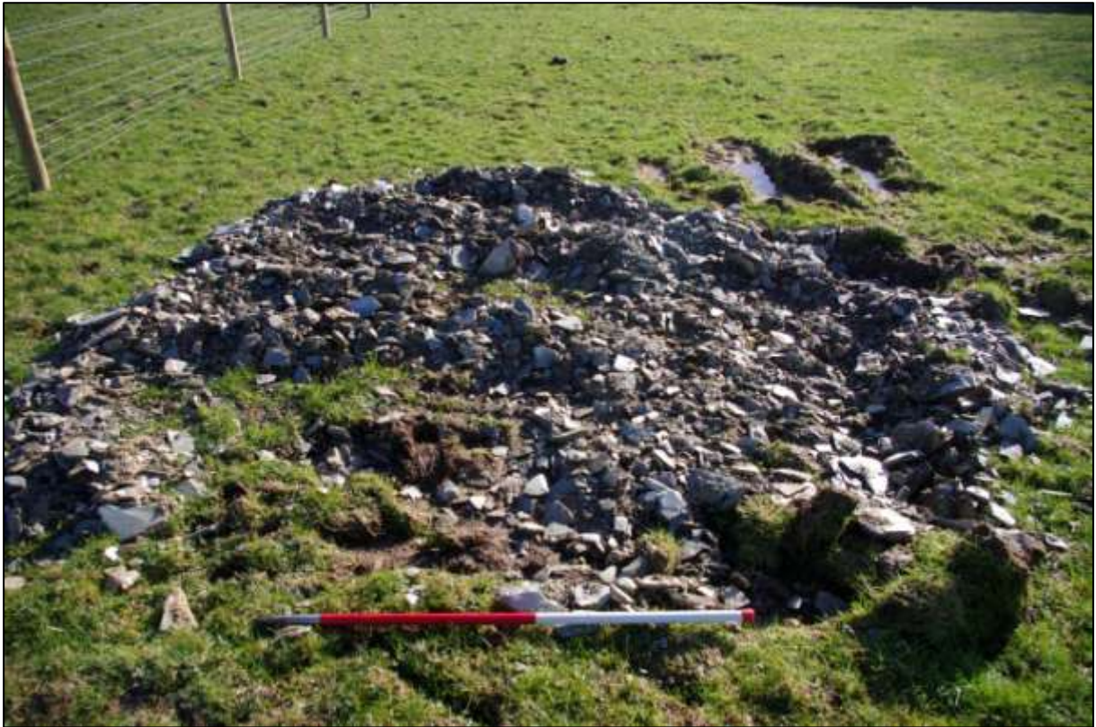
THE GEOTECHNICAL TEST PIT PART WAY ALONG THE NORTH-EASTERN BOUNDARY OF THE SITE (SCALE 1M).
