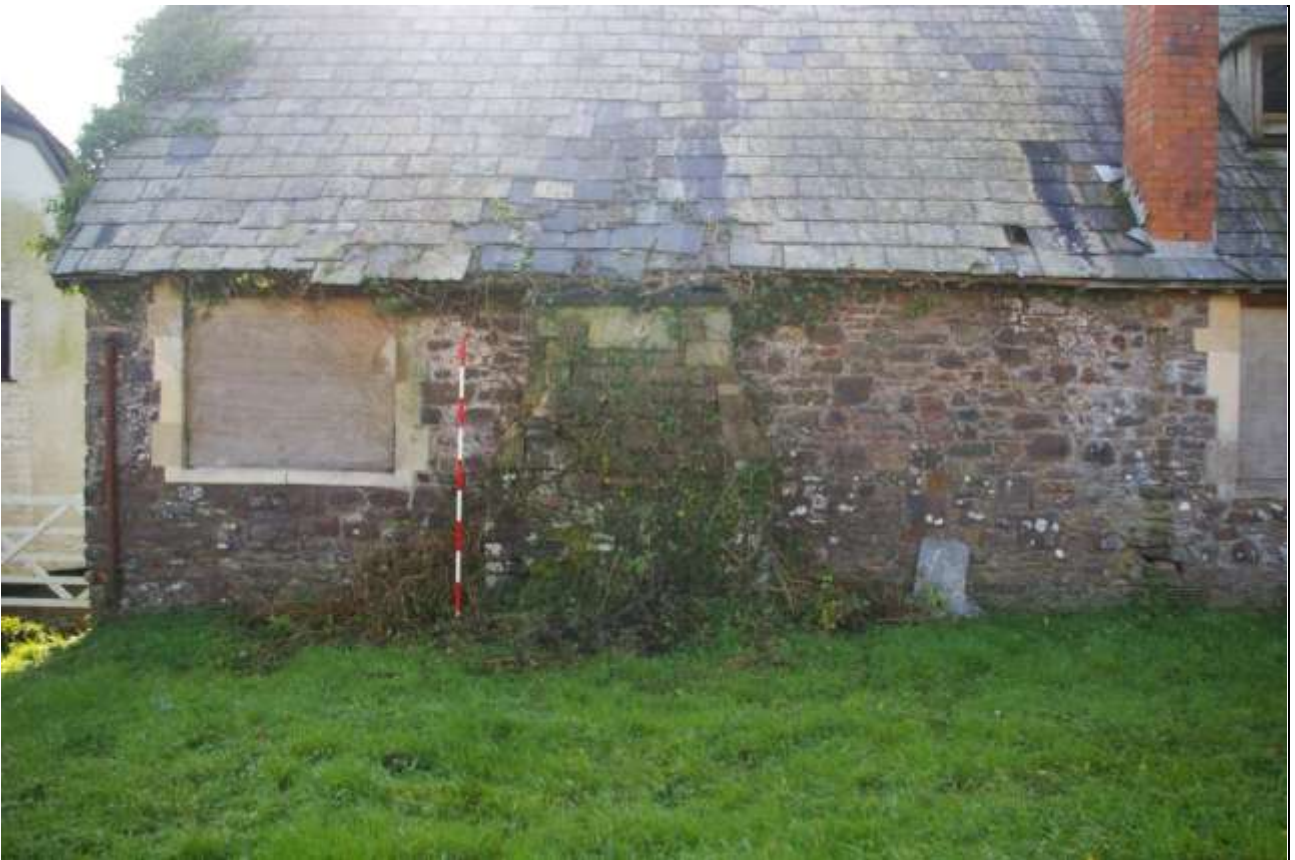
CHIMNEY INSERTED INTO THE NORTH ELEVATION OF THE SCHOOL HOUSE, VIEWED FROM THE NORTH (2M SCALE).
