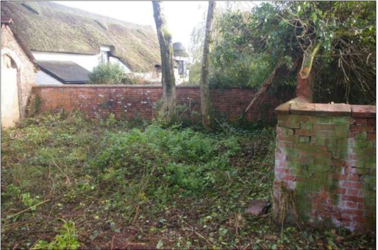
BRICK BOUNDARY WALL DEFINING FORMER PLAYGROUND AREA, VIEWED FROM THE SOUTH-WEST (NO SCALE).
