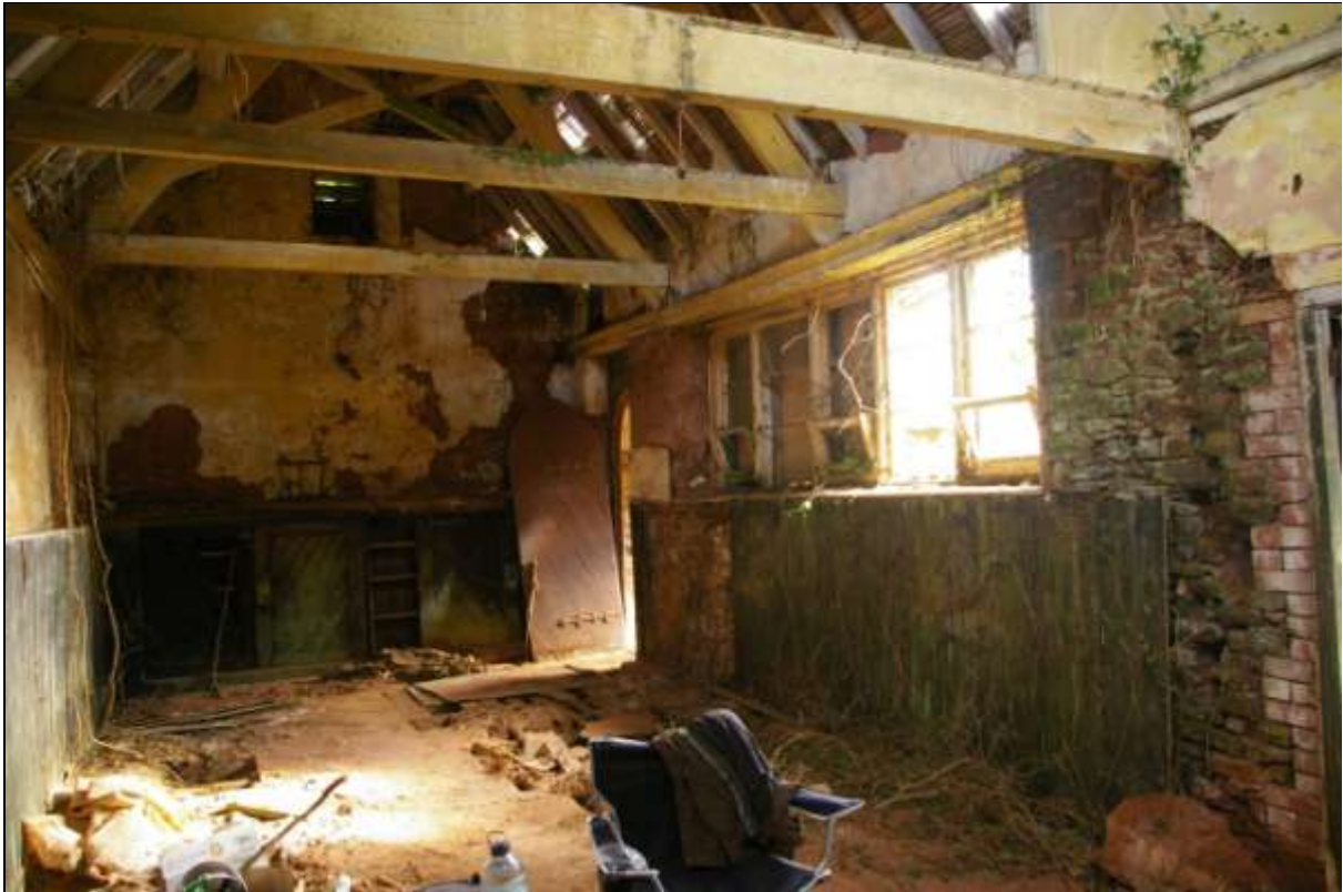
FIGURE 5: GENERAL SHOT OF THE INTERIOR OF THE SCHOOL ROOM, VIEWED FROM THE SOUTH-WEST (NO SCALE).
