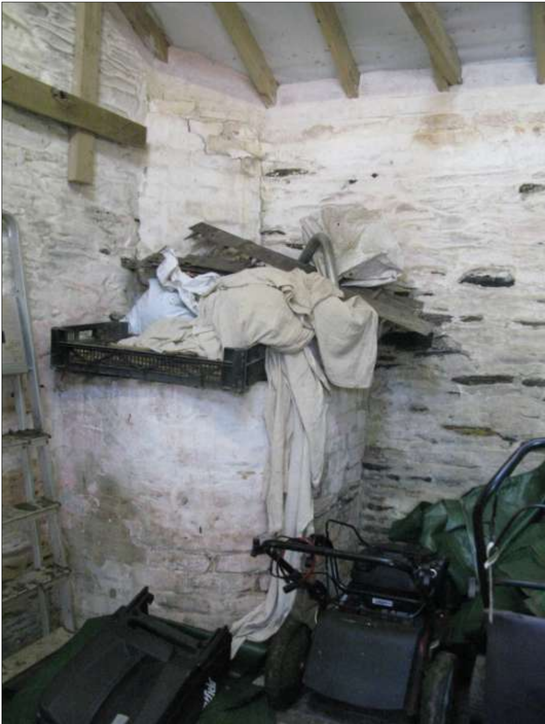
The brick-built boiler in the south-east corner of the south-range, back-to-back with the brick-built hearth; from the north, north-west
