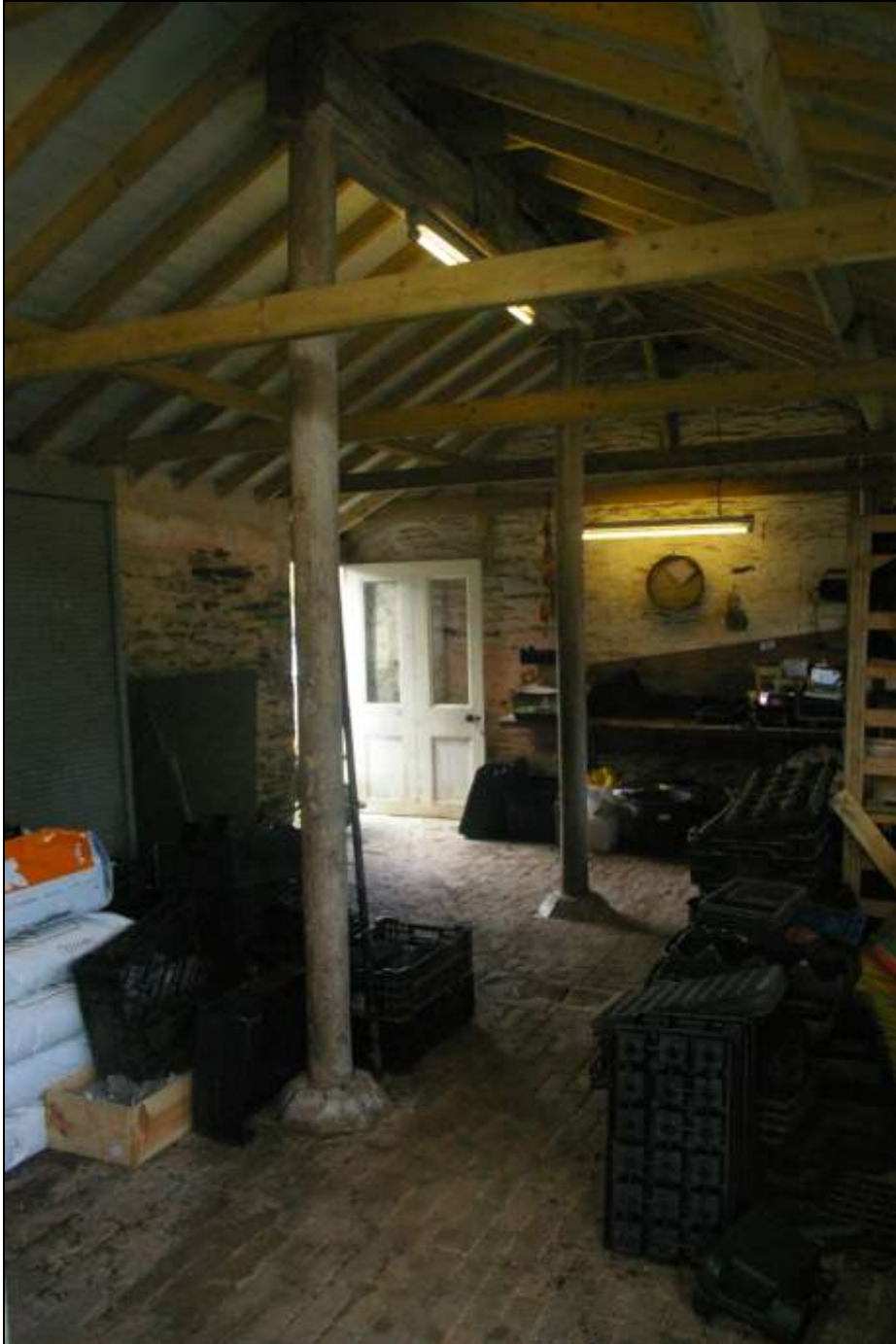
The interior of the large room, to the east end of the south range with the fitted timber frame and brick paved floor and drain; from the east, north-east
