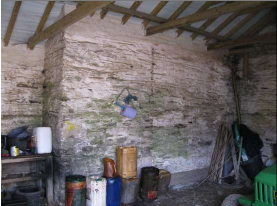
Block of earlier masonry, enclosed within the west end of the south range; from the north-east.
