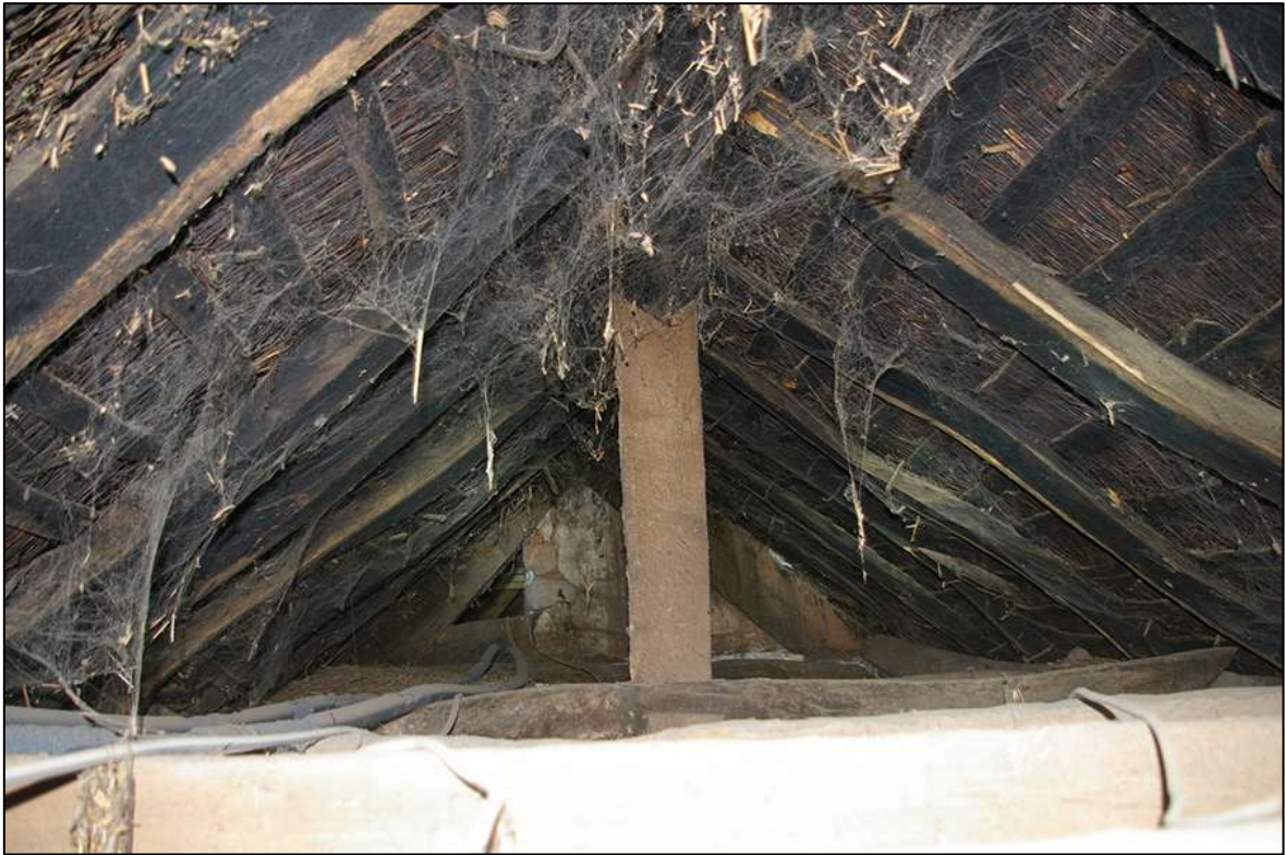
FIGURE 19: VIEW ABOVE THE CEILING JOISTS IN R6 AND R7/R8 TO THE AXIAL STACK; VIEWED FROM THE SOUTH-EAST.
