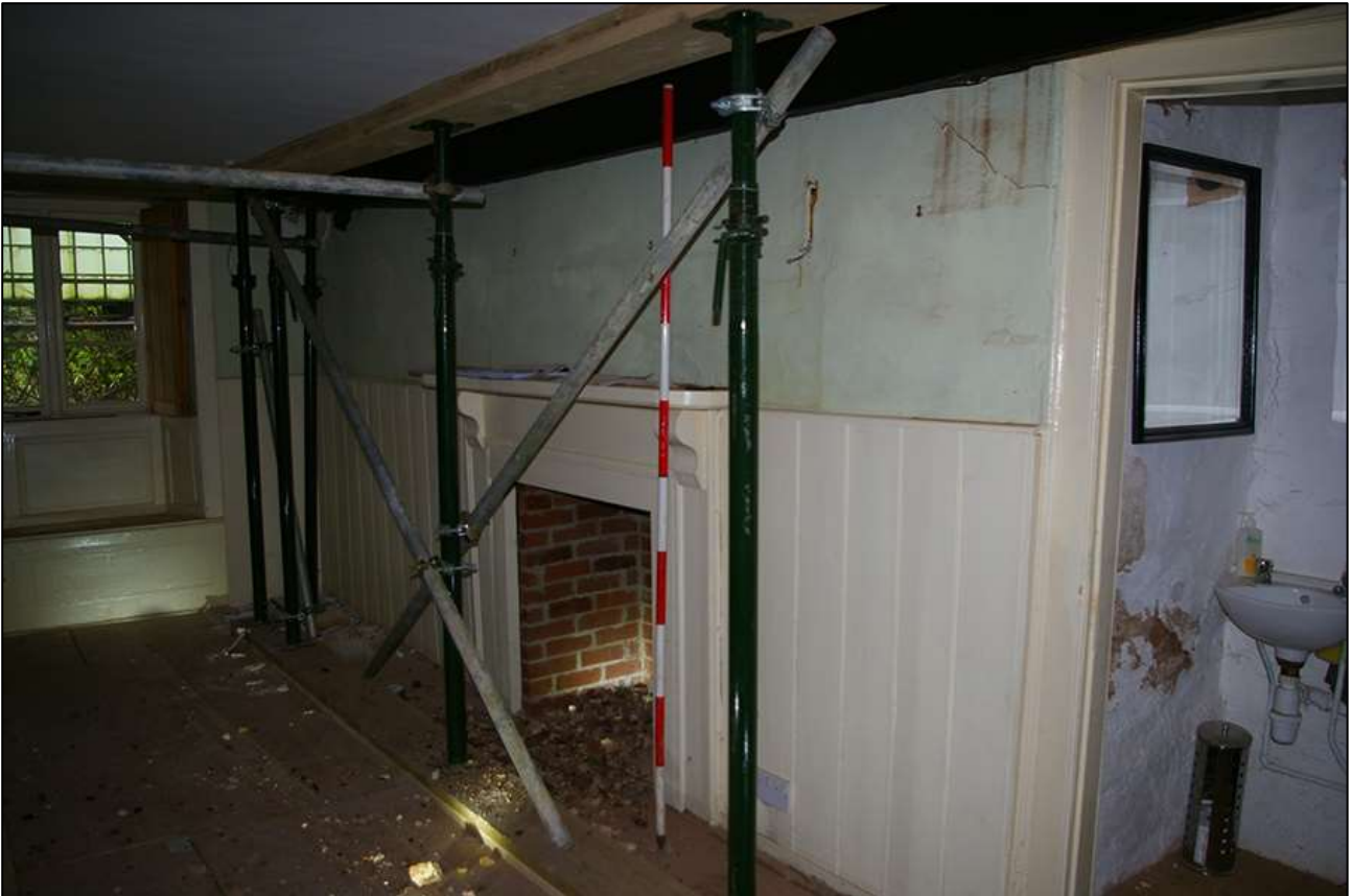
31. R2; FP2 PRIOR TO WORK COMMENCING. VIEWED FROM THE WEST (SCALE 2M).
