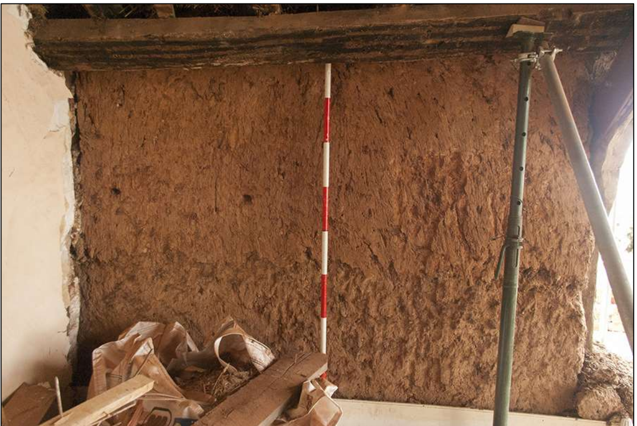
94. R6; DETAIL OF THE NORTH-EAST WALL SHOWING THE RAISE IN THE COB. VIEWED FROM THE SOUTH-WEST (SCALE 2M).
