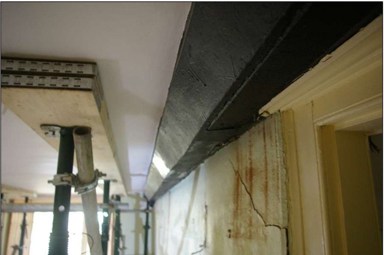
32. R2; DETAIL OF THE CHAMFERED BEAM ABOVE FP2; VIEWED FROM THE SOUTH-WEST.
