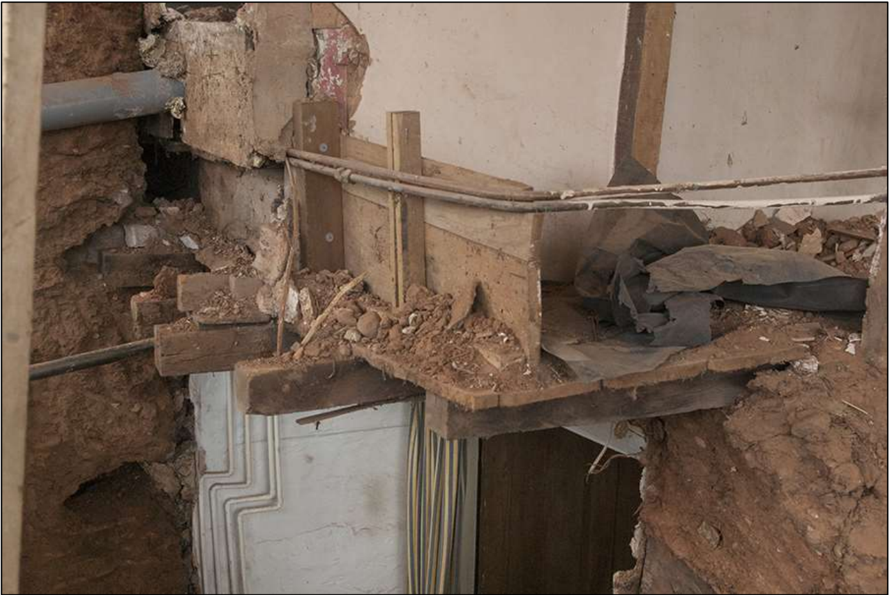
100. R6; THE HANGING FLOOR OF THE ALCOVE (GARDEROBE?) TO THE WEST OF THE GABLE STACK, VIEWED FROM THE EAST.
