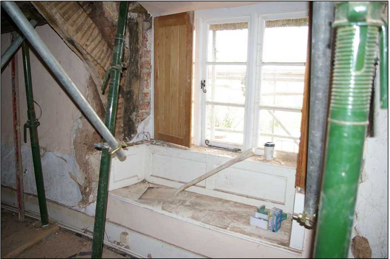
54. AS ABOVE; SHOWING THE FOOT OF THE FAILED TRUSS BLADE. VIEWED FROM THE SOUTH.
