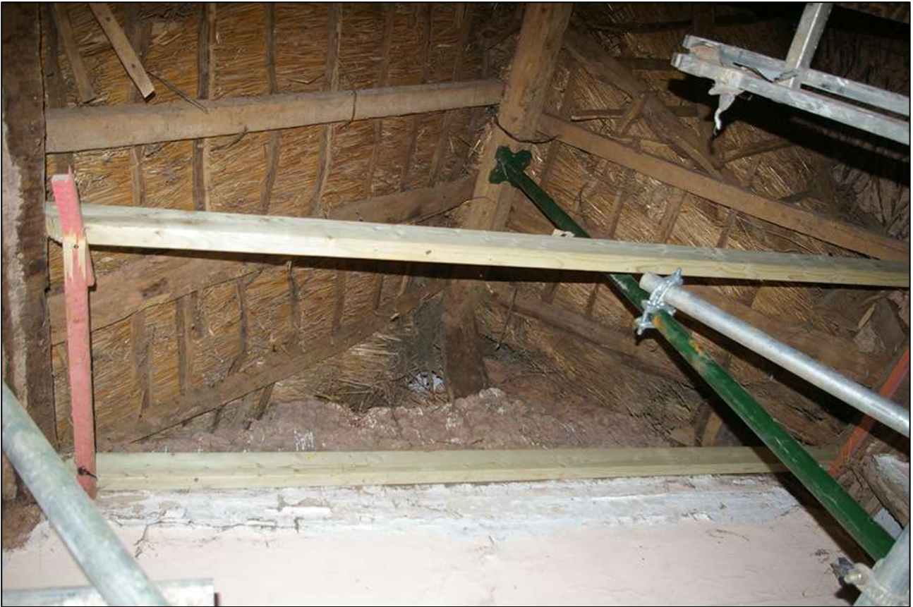
120. R6; THE APEX OF THE ROOF ABOVE THE GABLE END STACK. VIEWED FROM THE NORTH-WEST.
