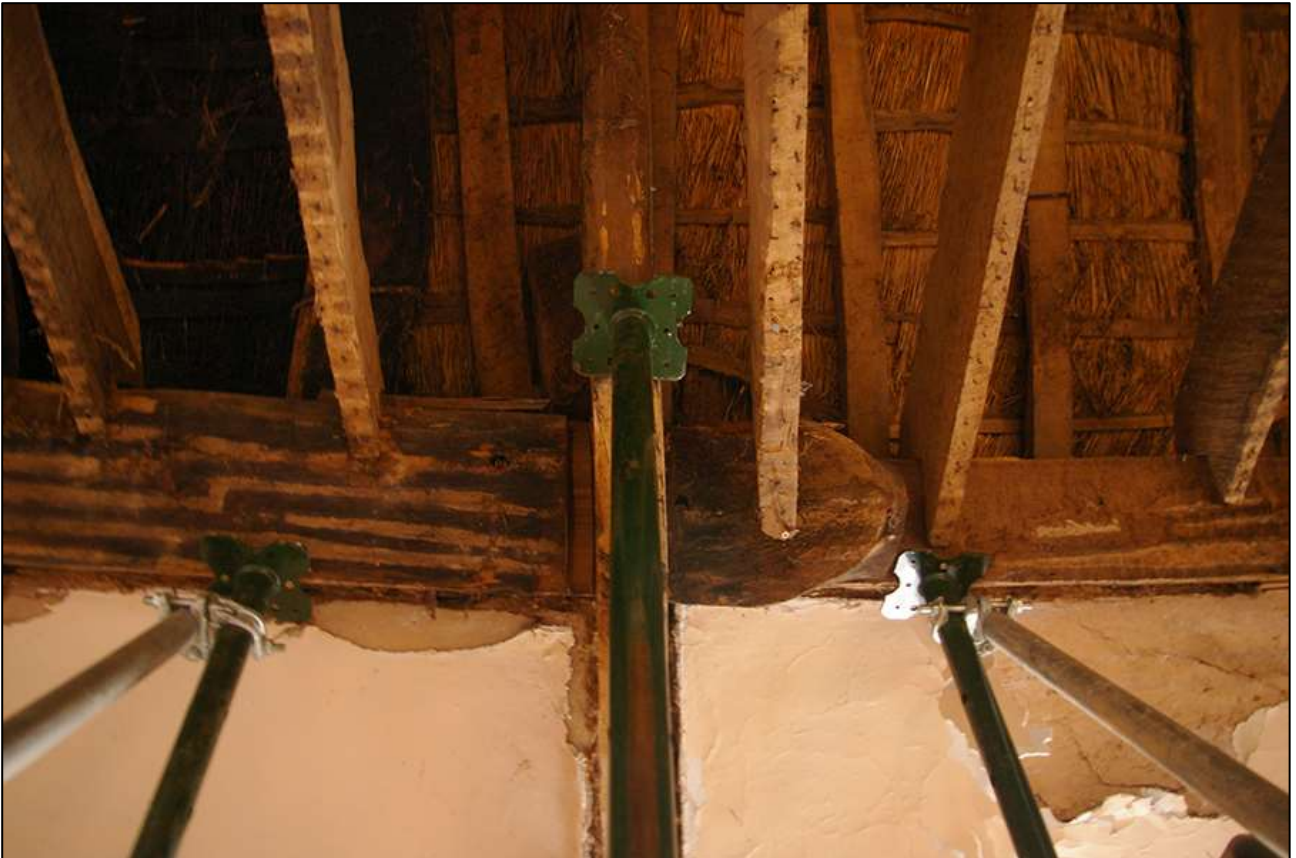
116. R6; THE UNDERSIDE OF THE FAILED TRUSS SHOWING THE JUNCTION WITH THE SMOKE-BLACKENED ROOF (LEFT) AND LATER, UNSTAINED ROOF (RIGHT); VIEWED FROM THE SOUTH-WEST.
