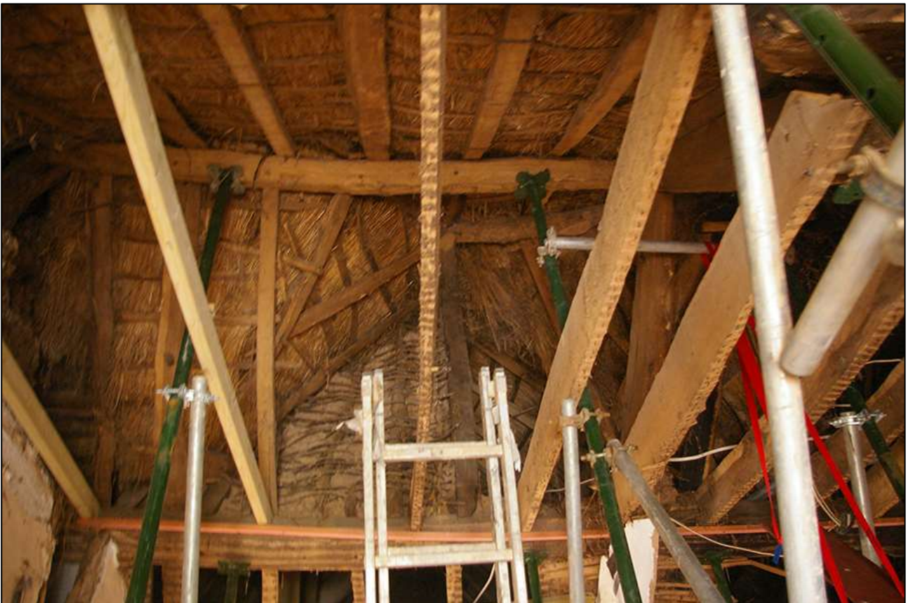
121. R6; THE SOUTH-WEST PITCH OF THE 17 TH CENTURY (UNSTAINED) ROOF SHOWING THE RELATIONSHIP WITH THE ROOF OF THE WING. VIEWED FROM THE NORTH-EAST. NOTE THE CRUDE WITHY-WITH-COB INFILL.
