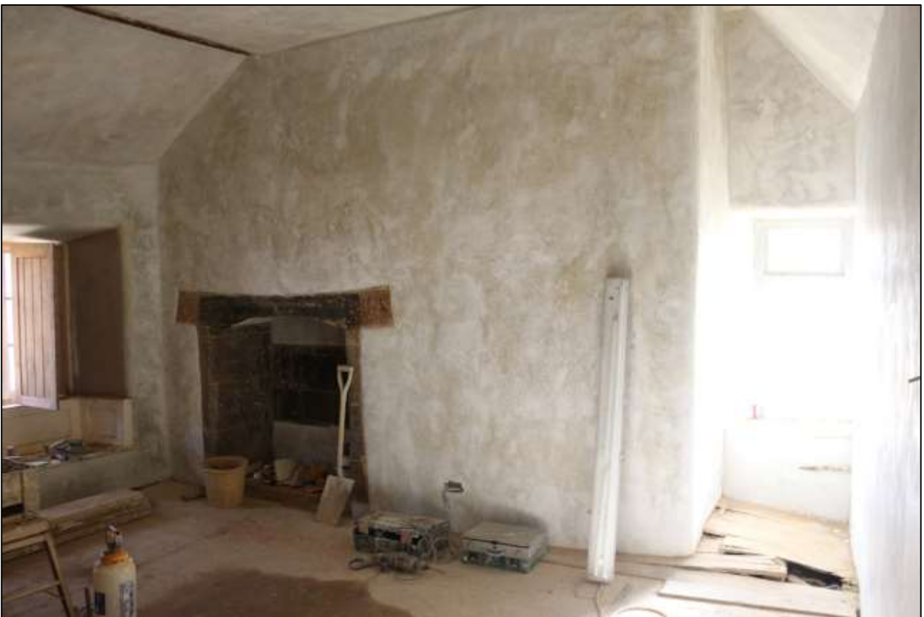
136. R6; VIEW OF THE GABLE AND FP4 AFTER REMEDIAL WORKS HAD BEEN COMPLETED. VIEWED FROM THE NNW.
