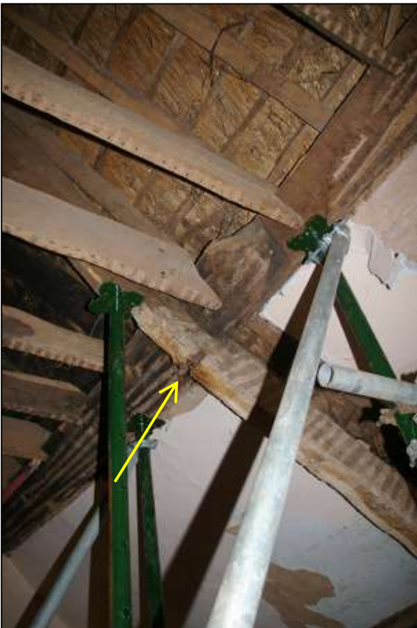
113. AS ABOVE; DETAILED OF THE FAILED TRUSS. VIEWED FROM THE SOUTH-SOUTH-EAST.
