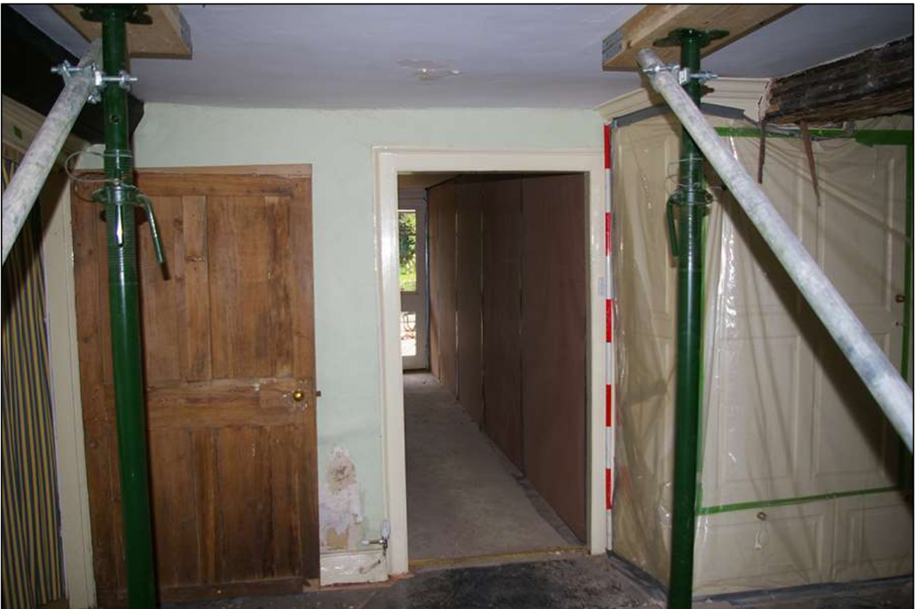
24. R2; SHOWING D2, WITH THE OPEN D3 TO THE LEFT AND 18 TH CENTURY CUPBOARD TO RIGHT; VIEWED FROM THE NORTH-EAST (SCALE 2M).
