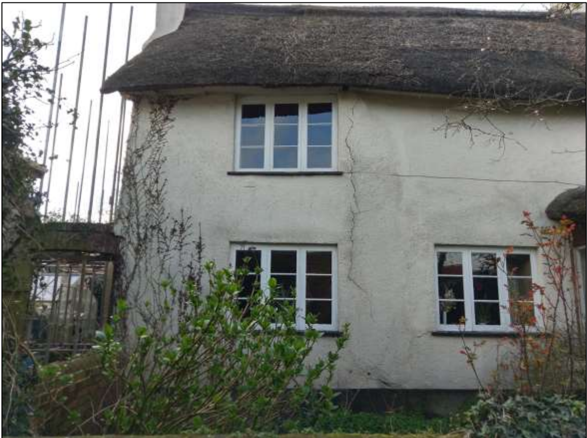
FIGURE 7: THE SOUTH END OF THE NORTH-EAST ELEVATION; THE BREAK OF BUILD TO THE RIGHT OF THE WINDOWS IS CLEARLY VISIBLE; VIEWED FROM THE NORTH-EAST (PHOTO SUPPLIED BY COB SOLUTIONS).
