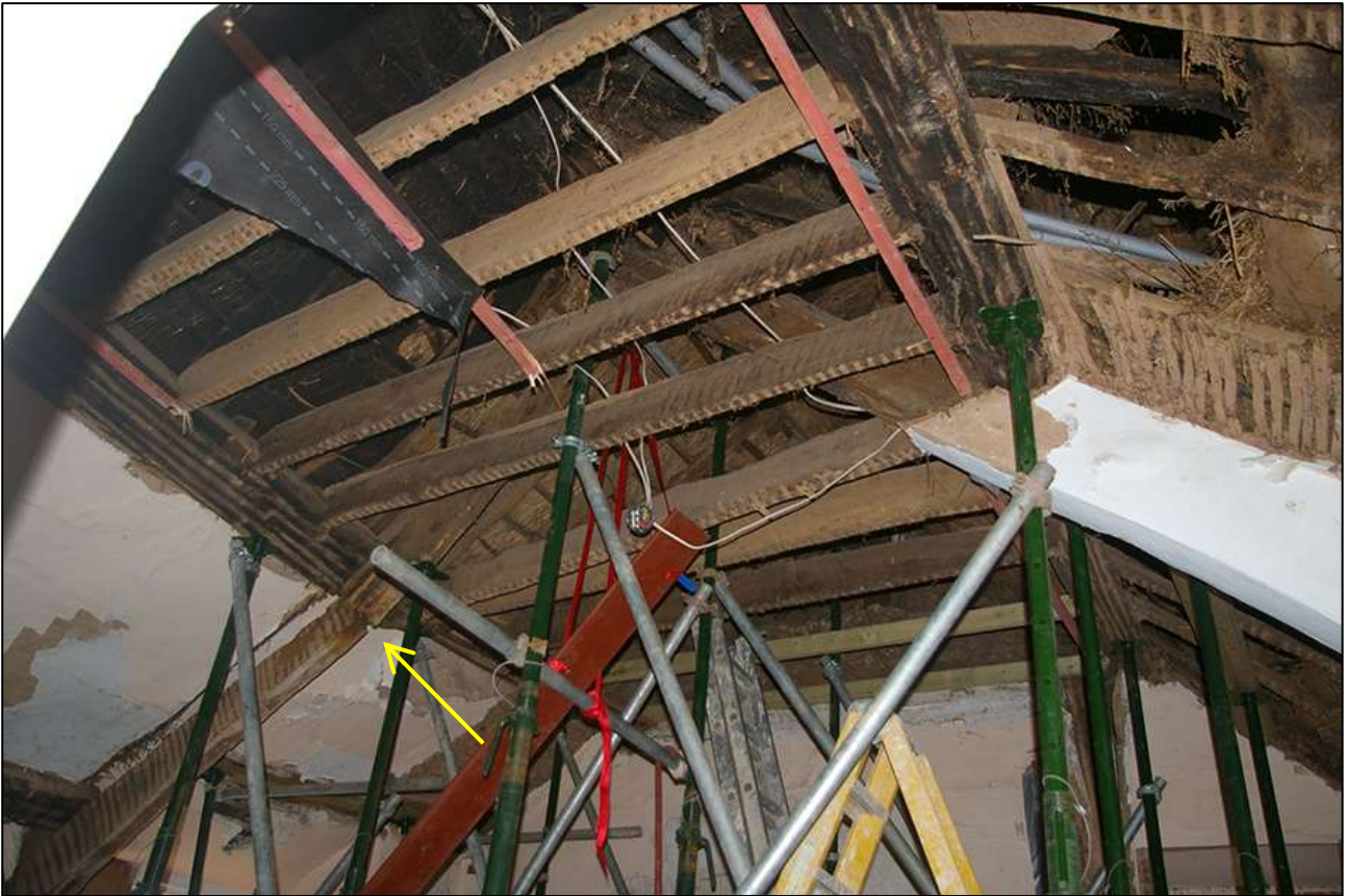
109. R6; SHOWING THE ROOF STRUCTURE AND FAILED TRUSS (INDICATED); VIEWED FROM THE WEST.
