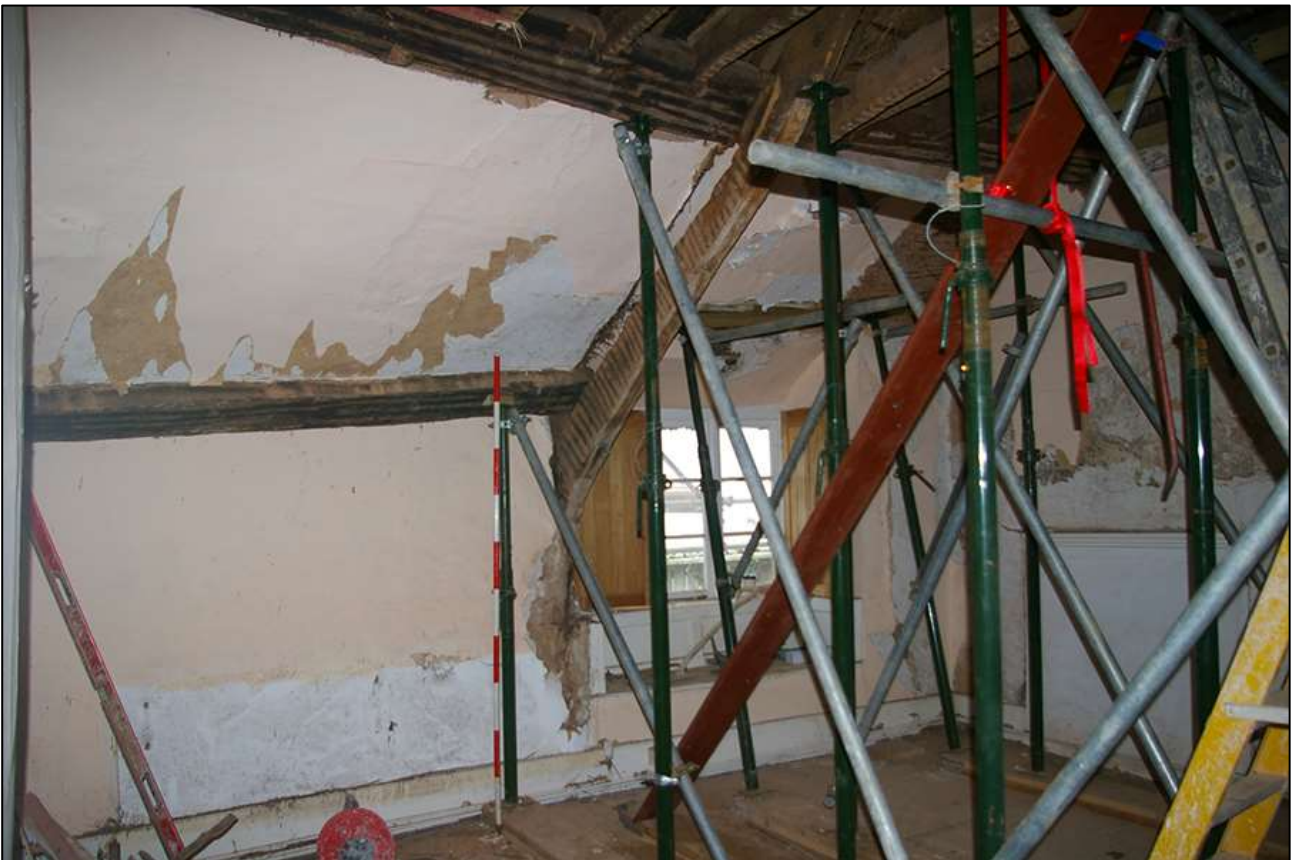
55. R6; VIEWED FROM THE WEST. SHOWING THE FAILED TRUSS BLADE (SCALE 2M).
