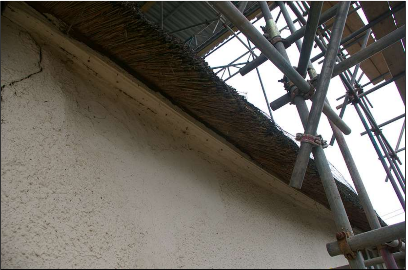
5. DETAIL OF THE MOULDED WALLPLATE ALONG THE NORTH-EAST ELEVATION; VIEWED FROM THE SOUTH.
