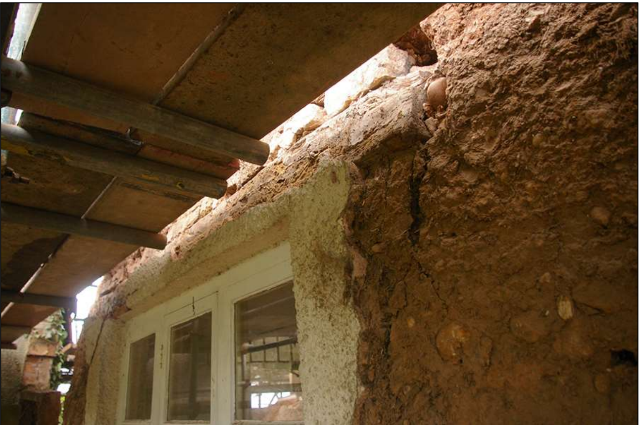
88. AS ABOVE; DETAIL OF THE LINTEL OVER W2; VIEWED FROM THE NORTH.
