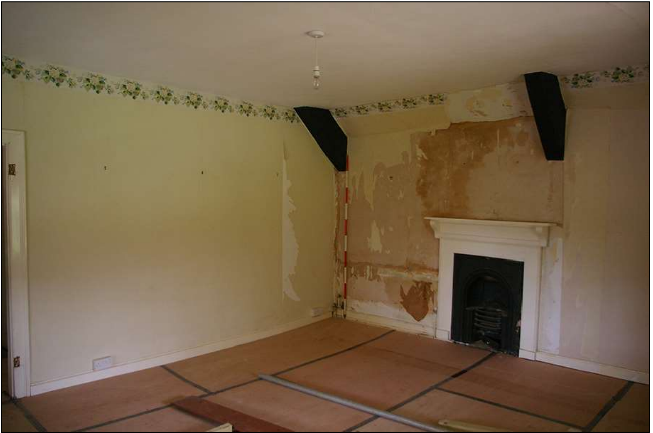
42. R4; VIEWED FROM THE WEST. SHOWING FP3 AND THE TWO TRUSS FEET (SCALE 2M).
