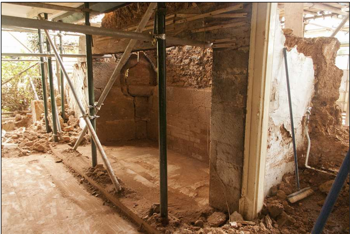
FIGURE 11: THE SAME VIEW AS WORKS PROGRESS, SHOWING THE EARLY 17 TH CENTURY HEARTH.
