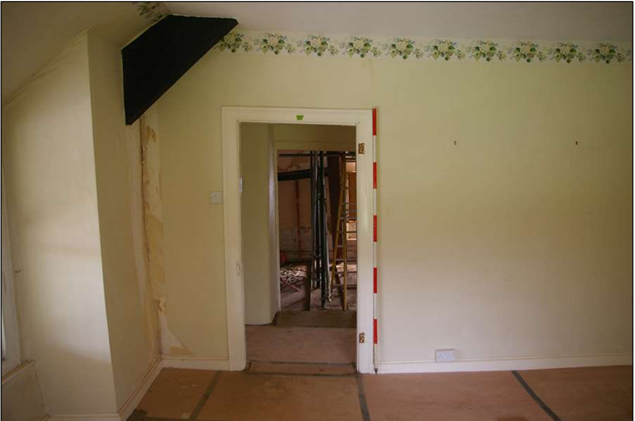
40. R4; LOOKING BACK THROUGH D6 INTO R3 WITH R6 BEYOND. VIEWED FROM THE SOUTH-WEST (SCALE 2M).
