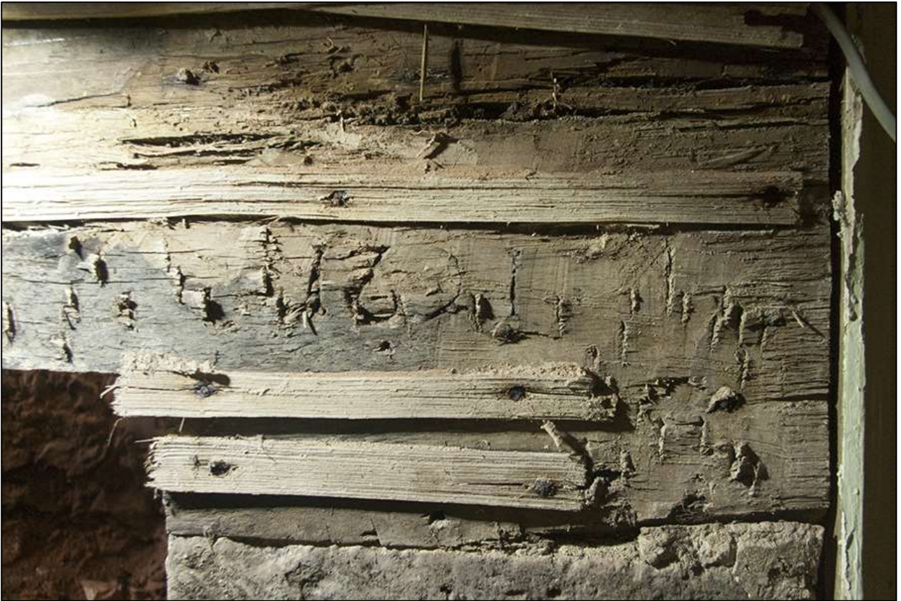
80. R2; DETAIL OF THE DATE (1621) SCORED INTO THE BRESSUMER BEAM OVER FP2; VIEWED FROM THE NORTH-WEST.
