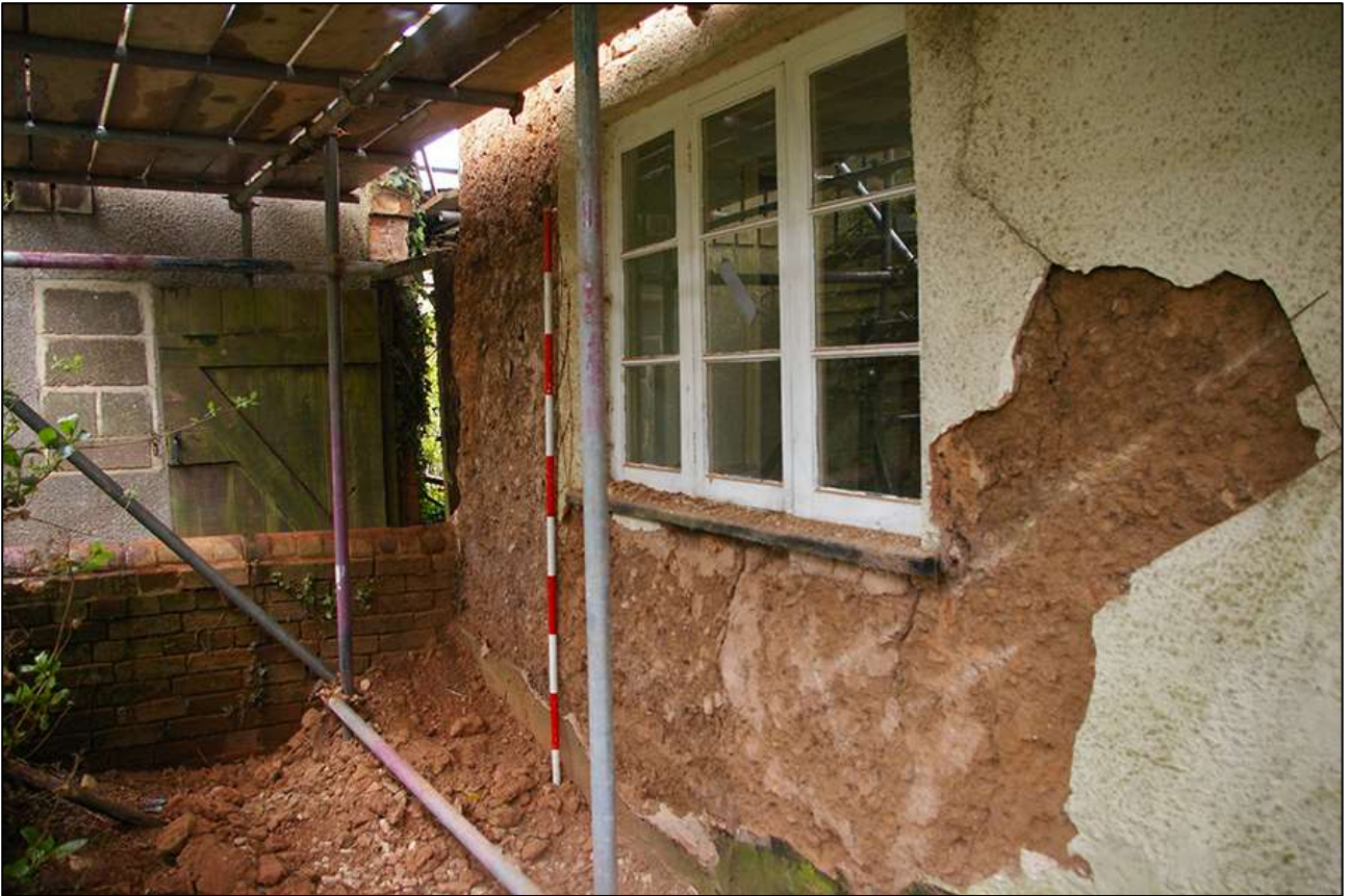
85. THE BASE OF THE NORTH-EAST ELEVATION FOLLOWING THE REMOVAL OF THE RENDER (W2); VIEWED FROM THE NORTH (SCALE 2M).
