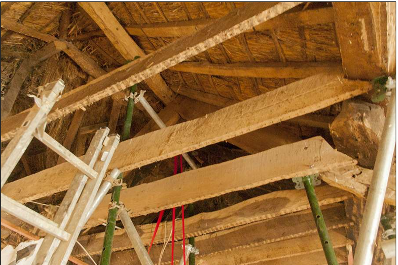
115. R6; DETAIL OF THE JOISTS AND THE ROOF STRUCTURE ABOVE CEILING LEVEL; VIEWED FROM THE SOUTH.
