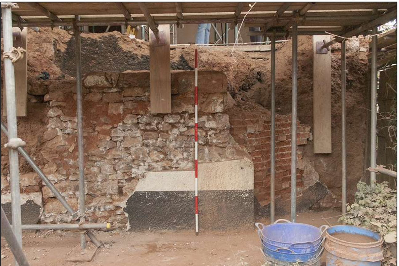
81. THE EXTERIOR ELEVATION OF FP2, SHOWING THE STONE RUBBLE BUILD; VIEWED FROM THE SOUTH-EAST (SCALE 2M).
