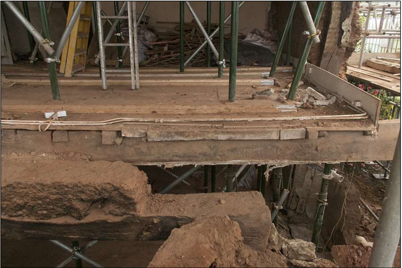
98. R6; THE TOP OF THE BRESSUMER BEAM OVER FP2 AND THE BACK OF THE CHAMFERED BEAM ABOVE; VIEWED FROM THE SOUTH-EAST.
