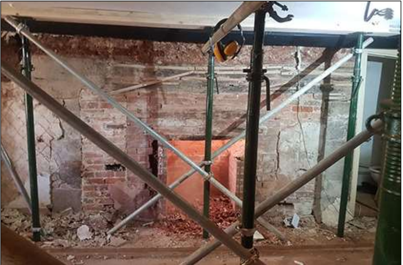
67. R6; FP2 STRIPPED OF PLASTER AND SHOWING THE SEVERAL PHASES OF BLOCKING. VIEWED FROM THE NORTH-WEST (PHOTO CREDIT: COB SOLUTIONS).
