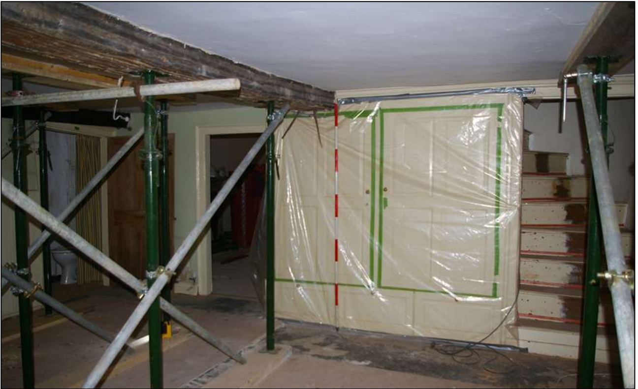
25. R2; VIEWED FROM THE EAST. SHOWING THE 18 TH CENTURY CUPBOARD AND STAIRS (R3) RISING TO THE FIRST FLOOR (SCALE 2M).
