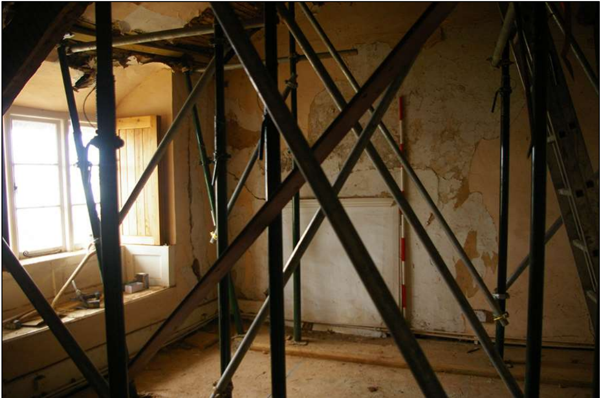
FIGURE 14: THE FIREPLACE IN R6, AS VIEWED THROUGH THE FOREST OF ACRO-PROPS; VIEWED FROM NORTH (SCALE 2M).
