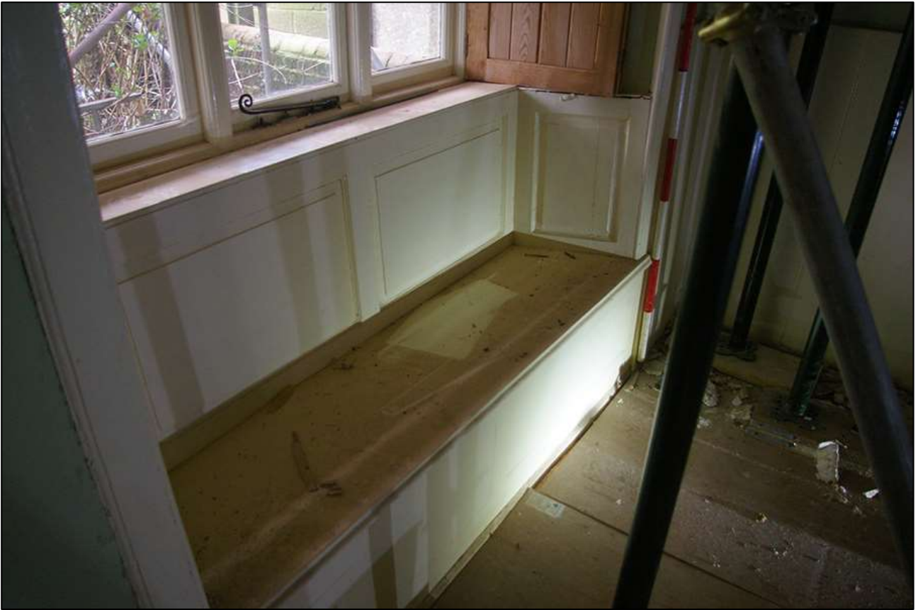
35. AS ABOVE, DETAIL OF THE WINDOW SEAT; VIEWED FROM THE NORTH (SCALE 2M).
