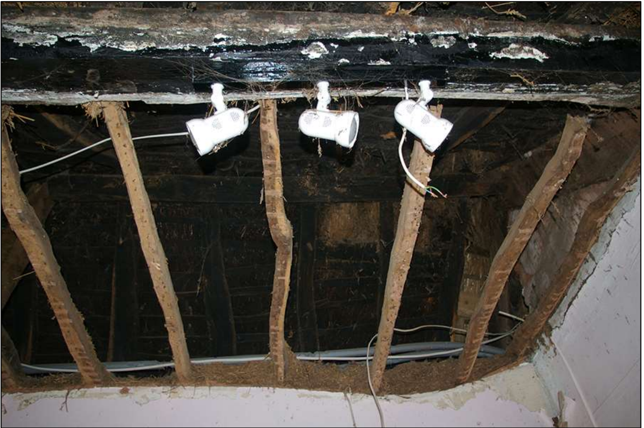
126. R7/R8; THE MEDIEVAL SMOKE-BLACKENED ROOF ABOVE CEILING LEVEL. VIEWED FROM THE NORTH-EAST.
