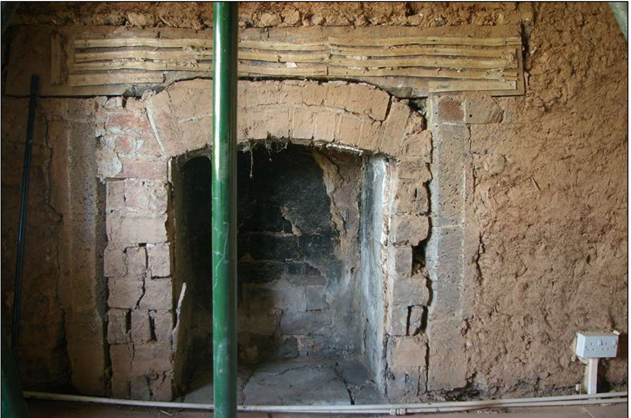
93. R6; DETAIL OF THE UNCOVERED 18 TH CENTURY FIREPLACE (FP4). VIEWED FROM THE NORTH-EAST.
