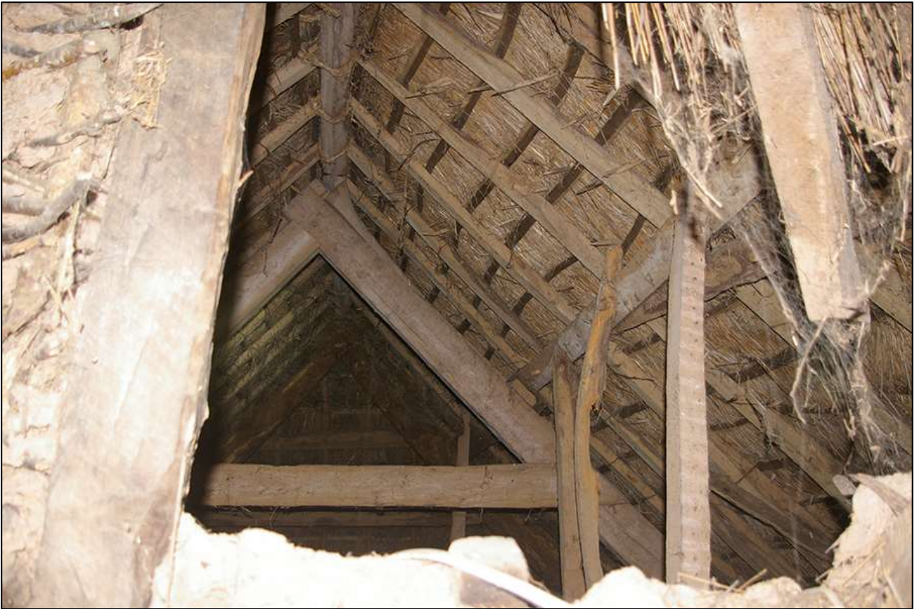
122. ABOVE R4; VIEW THROUGH TO THE 1860S ROOF STRUCTURE OF THE WING. VIEWED FROM THE NORTH-EAST.
