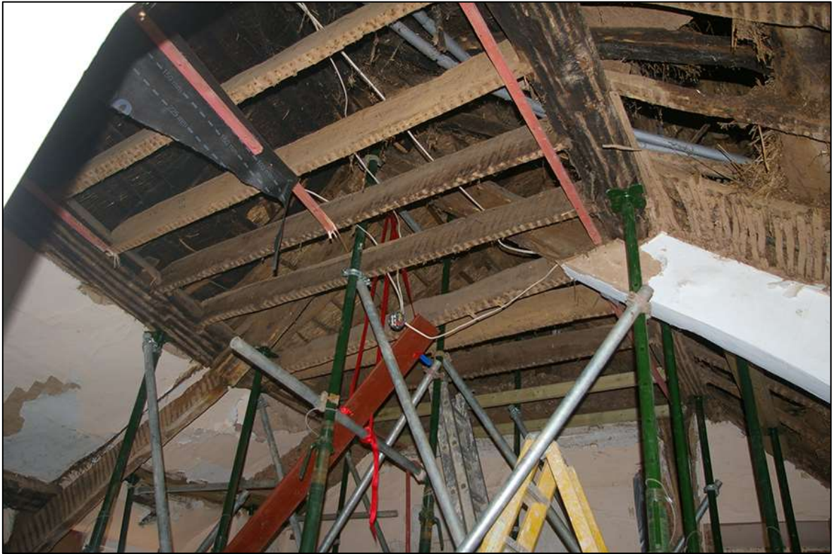
FIGURE 17: THE FAILED TRUSS BLADE IN THE 17 TH CENTURY TRUSS IN R6; VIEWED FROM THE NORTH.
