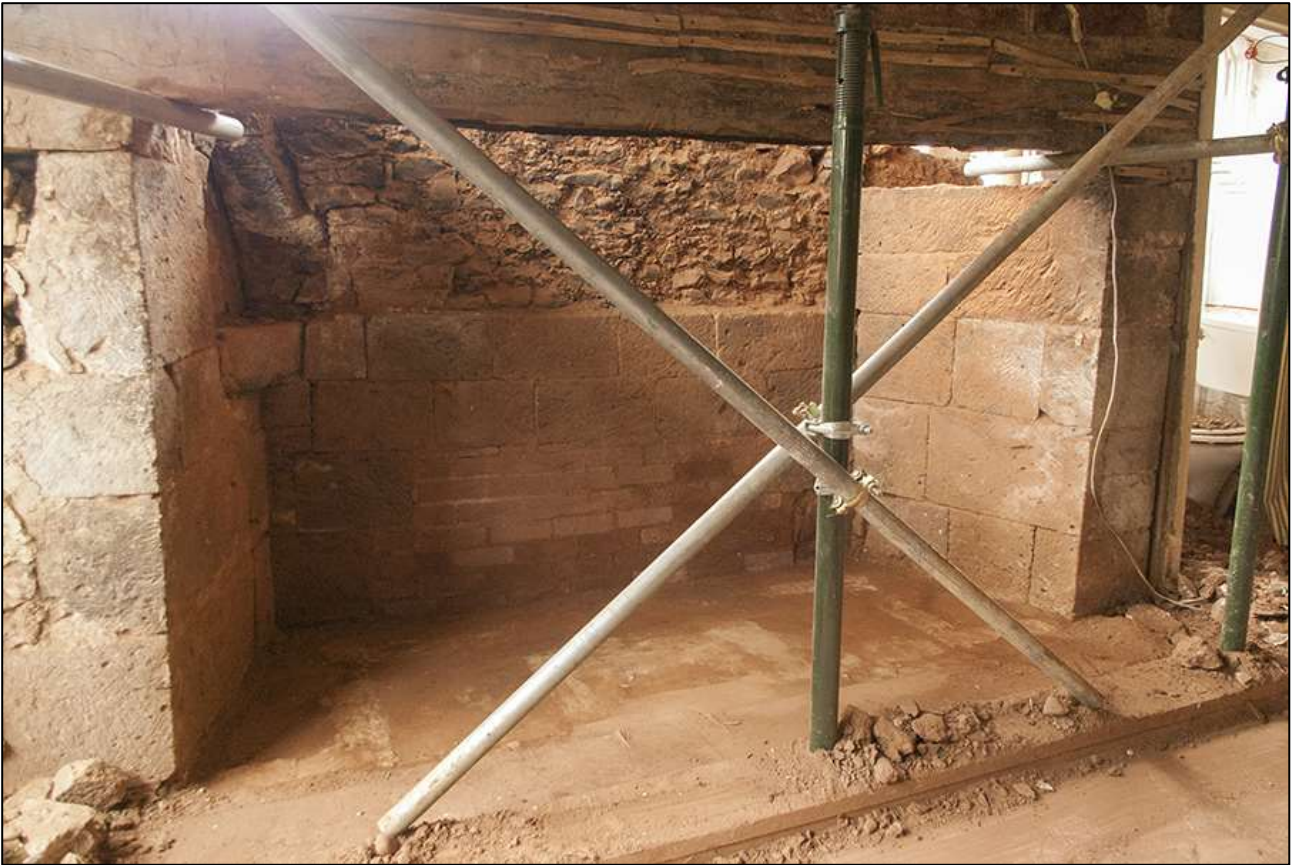
75. R2; SHOWING FP CLEARED OF ALL LATER BLOCKING MATERIAL. VIEWED FROM THE NORTH.
