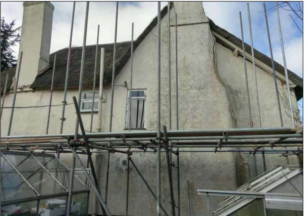
4. THE SOUTH-EAST ELEVATION OF THE MAIN RANGE; VIEWED FROM THE SOUTH-EAST (PHOTO CREDIT: COB SOLUTIONS)
