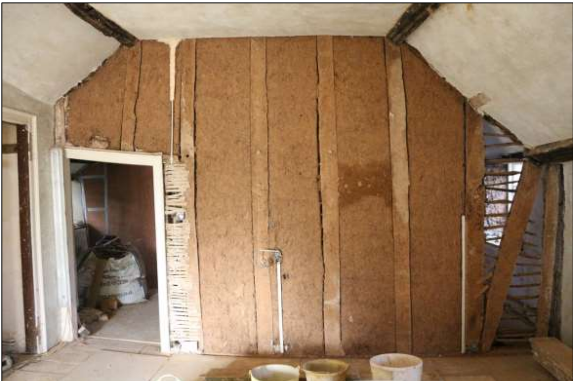
FIGURE 12: THE STUD AND COB WALL BETWEEN R6 AND R7/R8, WITH THE 18 TH CENTURY DOORWAY AWKWARDLY INSERTED TO THE LEFT; VIEWED FROM THE SOUTH-EAST.
