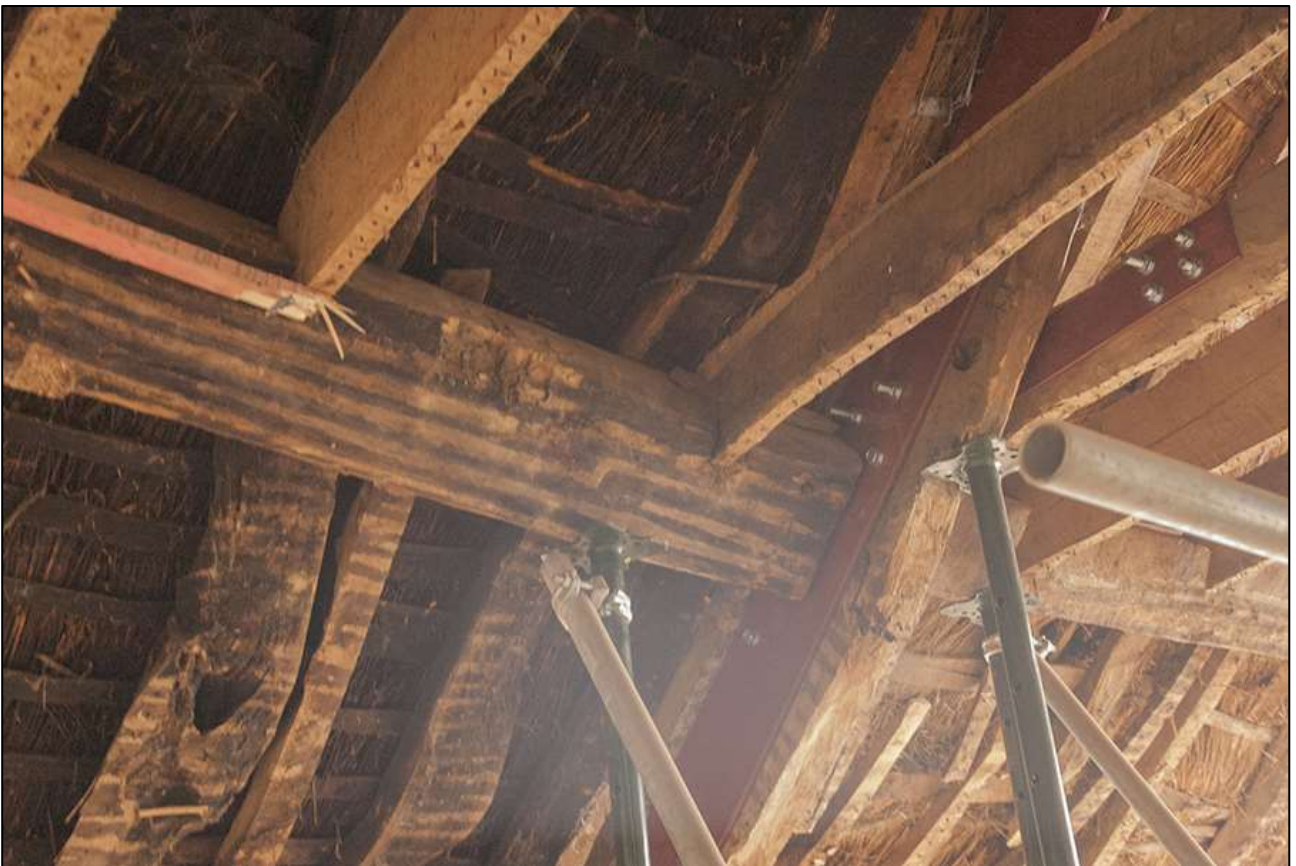
117. AS ABOVE; FOLLOWING THE REPAIR TO THE TRUSS BLADE. VIEWED FROM THE WEST. NOTE THE HEAVY MEDIEVAL PURLIN.
