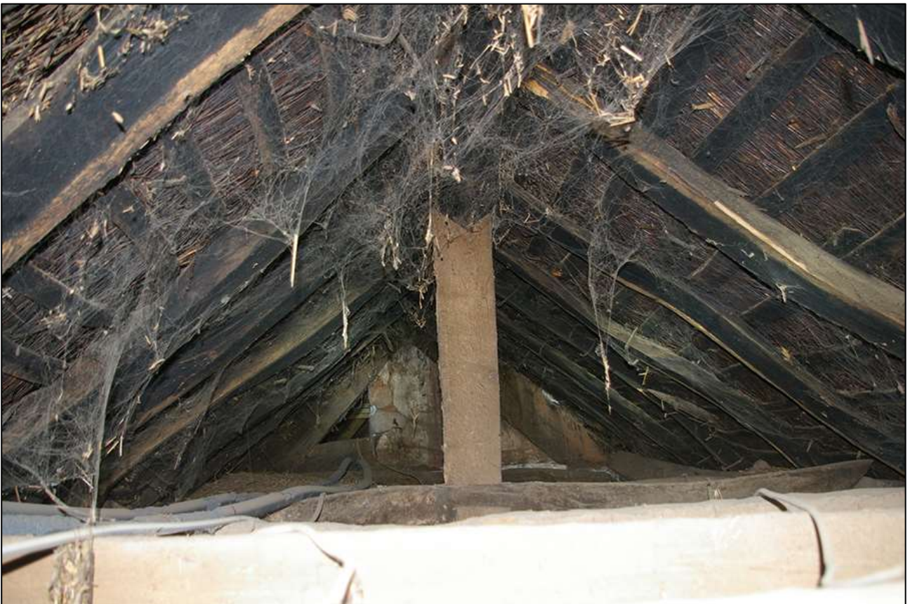
123. ABOVE R6/R7/R8; VIEW ABOVE CEILING LEVEL OF THE MEDIEVAL SMOKE-BLACKENED ROOF; VIEWED FROM THE SOUTH-EAST.
