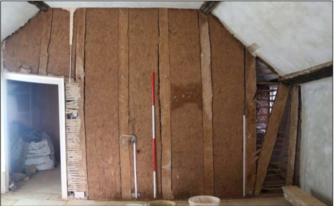
102. R6; THE PARTY WALL WITH R7/R8 STRIPPED OF PLASTER. VIEWED FROM THE SOUTH-EAST (SCALE 2M).
