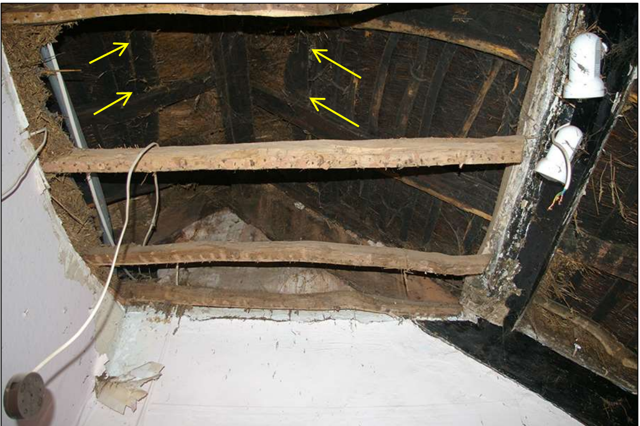
125. R8; THE APEX OF THE MEDIEVAL ROOF AND CRUCK TRUSS. VIEWED FROM THE SOUTH-EAST. THE REMAINS OF THE SMOKE LOUVRE ARE INDICATED.
