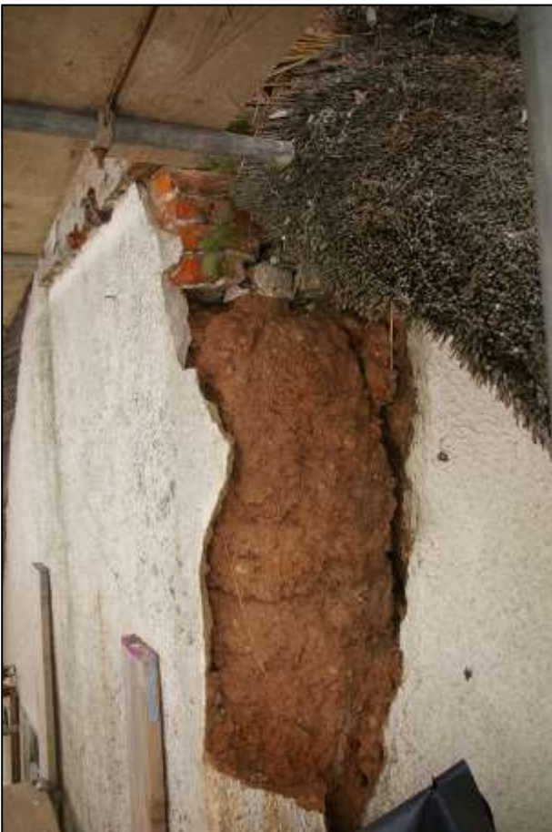
8. DETAIL OF THE STRUCTURAL CRACK DOWN THE SIDE OF THE GABLE END STACK; VIEWED FROM THE EAST.
