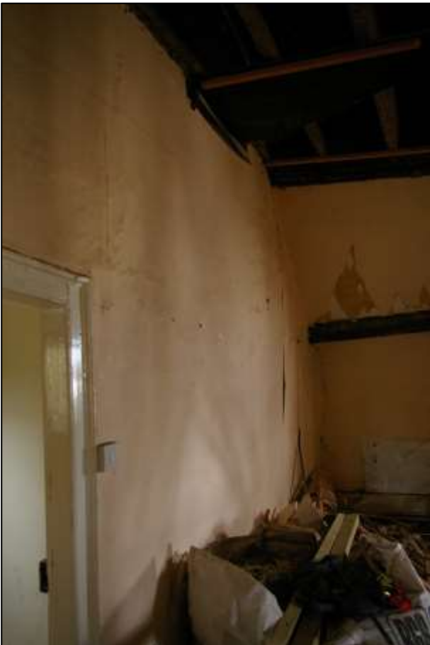
57. R6; THE PARTY WALL WITH R8 SHOWING ITS DEFORMATION. VIEWED FROM THE SOUTH-WEST.
