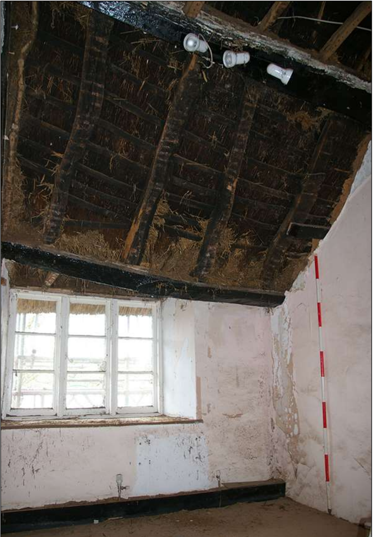
66. R8; DETAIL OF PART OF THE SMOKE-BLACKENED ROOF STRUCTURE ABOVE W10. VIEWED FROM THE SOUTH-WEST (SCALE 2M).
