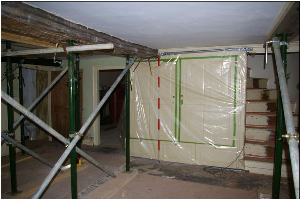
FIGURE 9: THE SOUTH-WEST WALL OF R2, WITH THE 18 TH CENTURY CUPBOARDS; VIEWED FROM THE NORTH-EAST (SCALE 2M).
