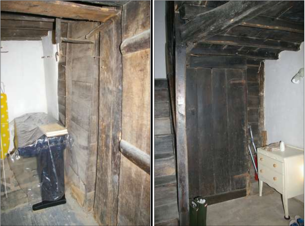
LEFT: STAIRHALL, UNDER THE STAIRS, SHOWING THE BACK OF THE CUPBOARD IN THE PARLOUR (S6); VIEWED FROM THE SOUTH. RIGHT: STAIRHALL, THE DOOR TO THE UNDERSTAIRS SPACE; VIEWED FROM THE SOUTH.
