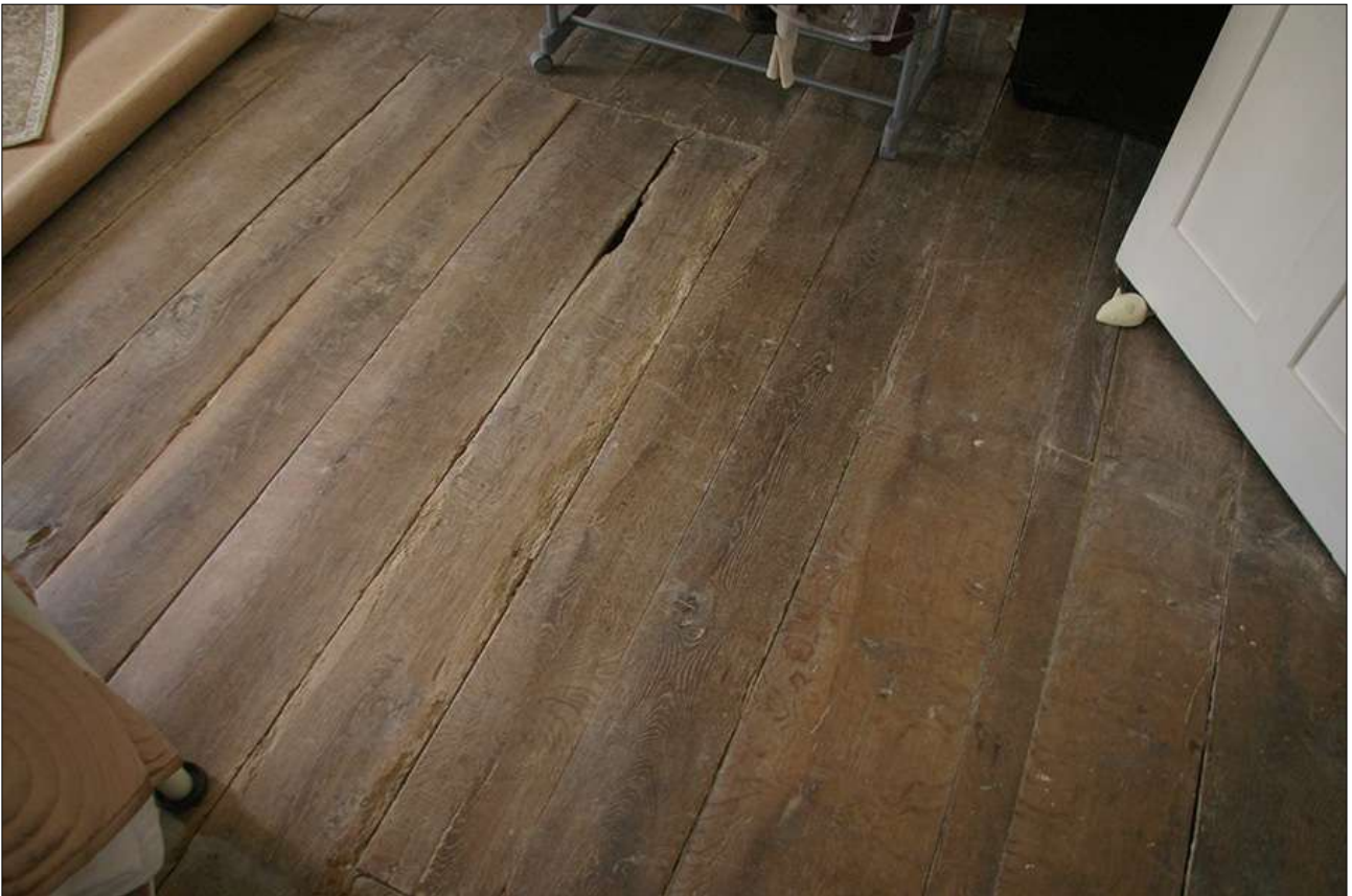
AS ABOVE, THE FLOORBOARDS JUST INSIDE THE DOOR; VIEWED FROM THE NORTH.
