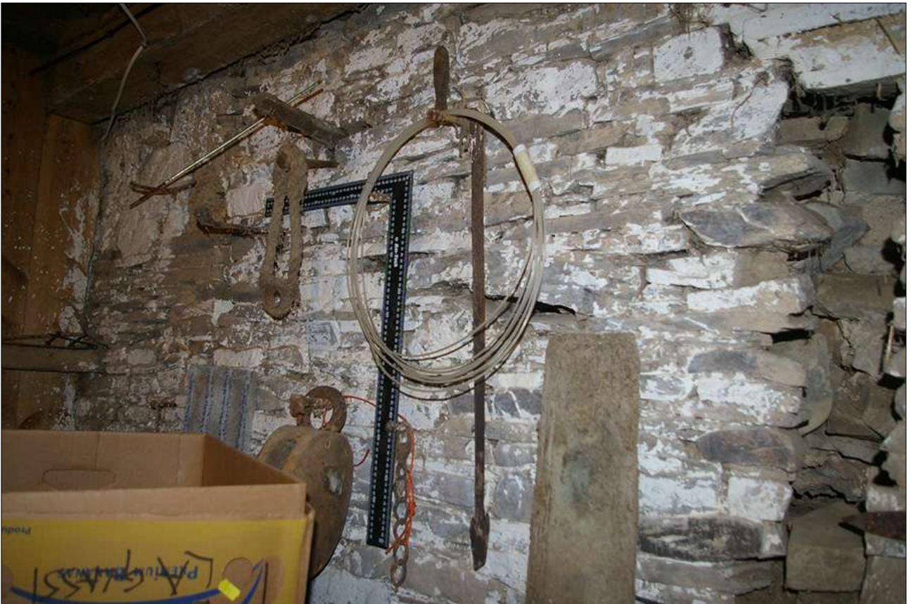
CROSS PASSAGE WEST END, SOUTH WALL, SHOWING BO3; VIEWED FROM THE NORTH.
