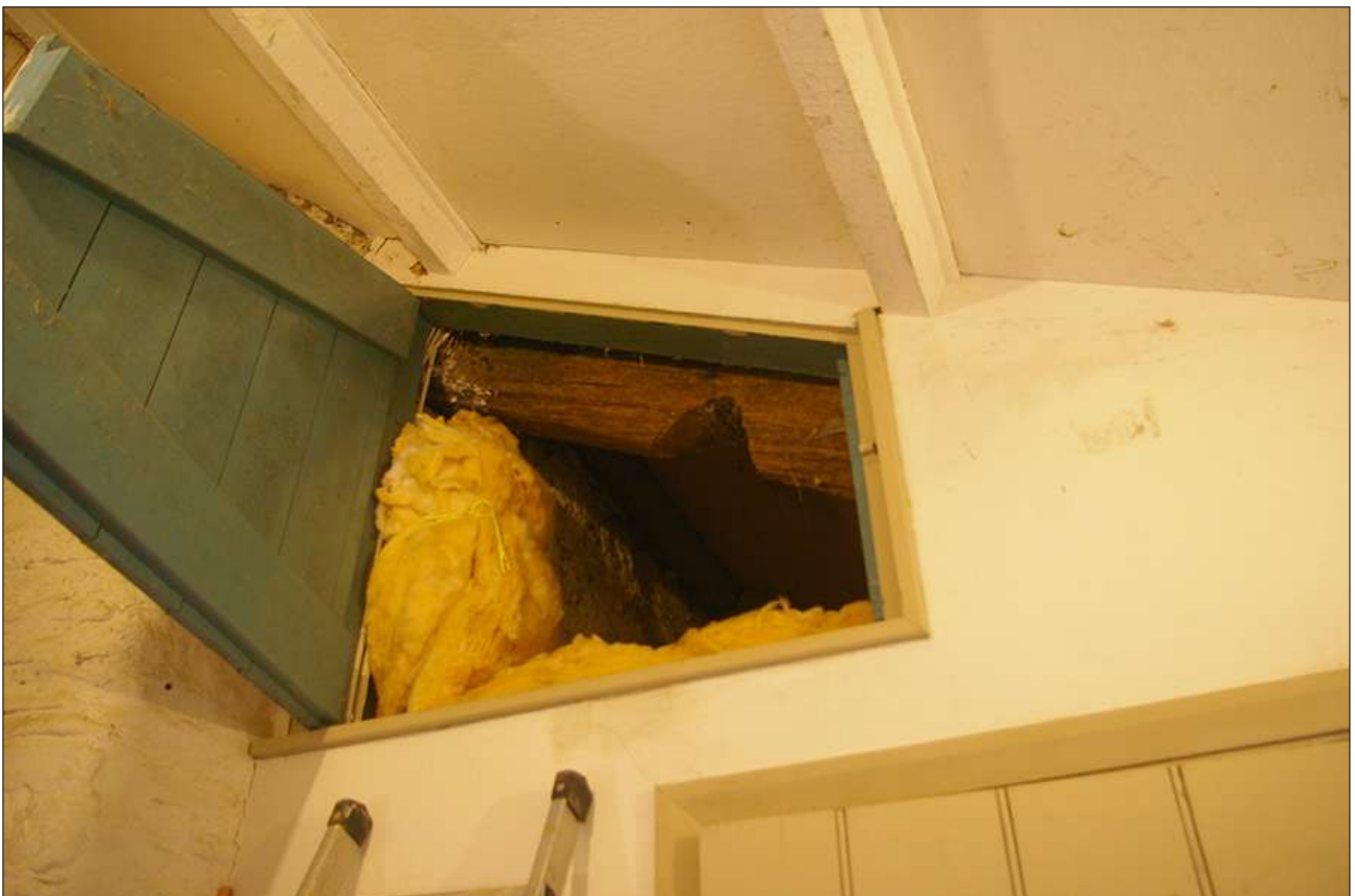
PUMP ROOM, SOUTH WALL STORAGE ABOVE PARTITIONED ROOM; VIEWED FROM THE NORTH.
