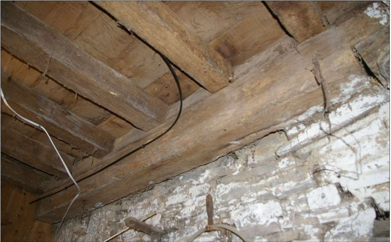
CROSS PASSAGE WEST END, SOUTH WALL, SHOWING THE EXPOSED JOISTS; VIEWED FROM THE NORTH.
