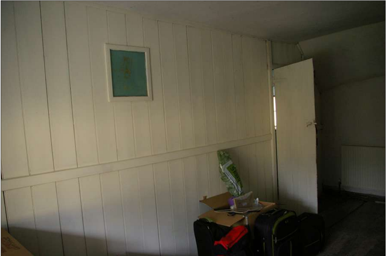
BEDROOM 3, THE 20 TH CENTURY PLANK PARTITION WALL WITH BEDROOM 4; VIEWED FROM THE NORTH-EAST.
