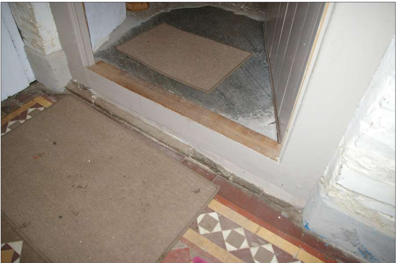
CROSS PASSAGE NORTH WALL, SHOWING THE THRESHOLD OF D2; VIEWED FROM THE SOUTH.
