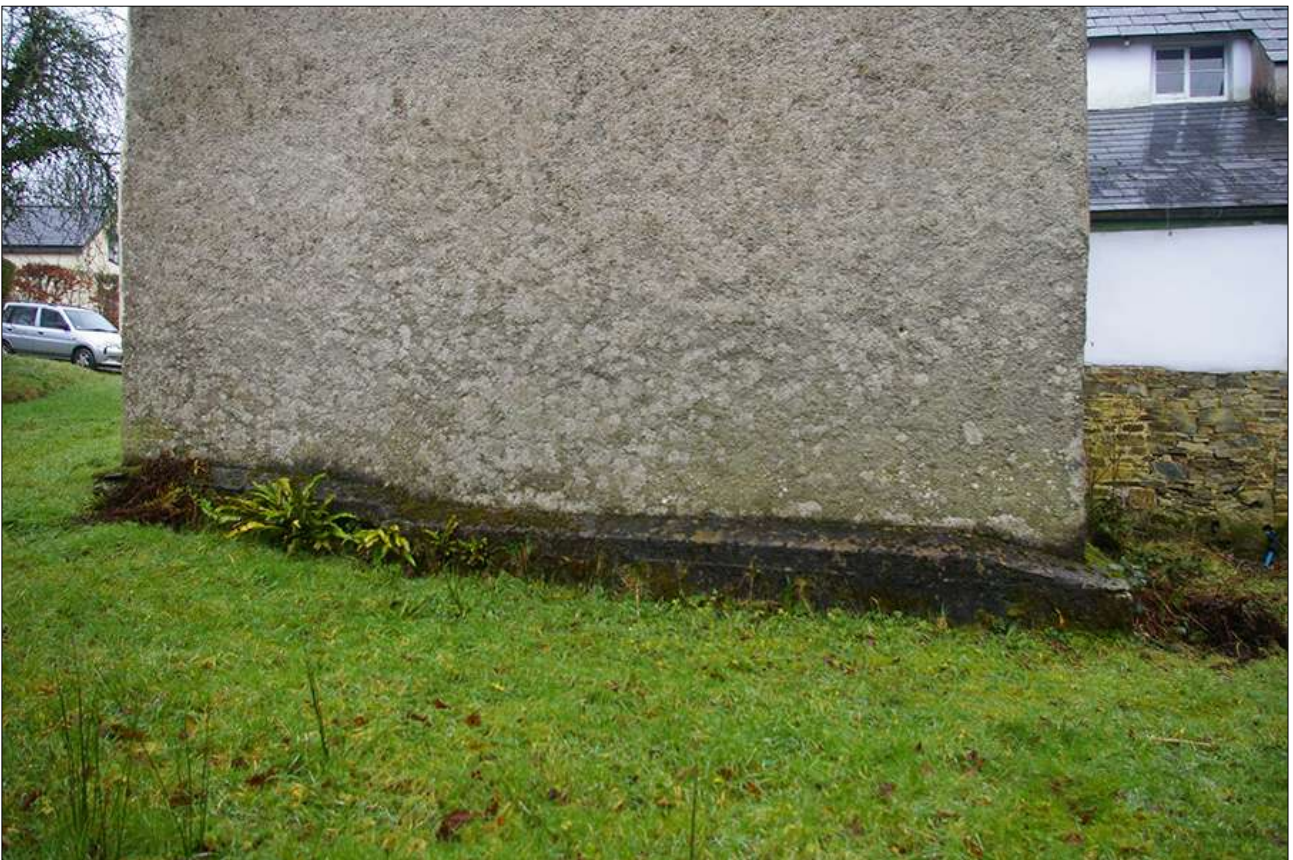
BASE OF THE WEST ELEVATION OF THE CROSSWING; VIEWED FROM THE WEST. NOTE THE CONCRETE PLINTH.
