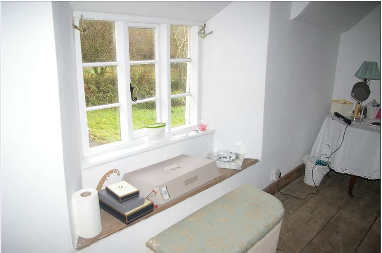
BEDROOM 2, THE WINDOW IN THE EAST WALL (W9); VIEWED FROM THE NORTH-WEST.
