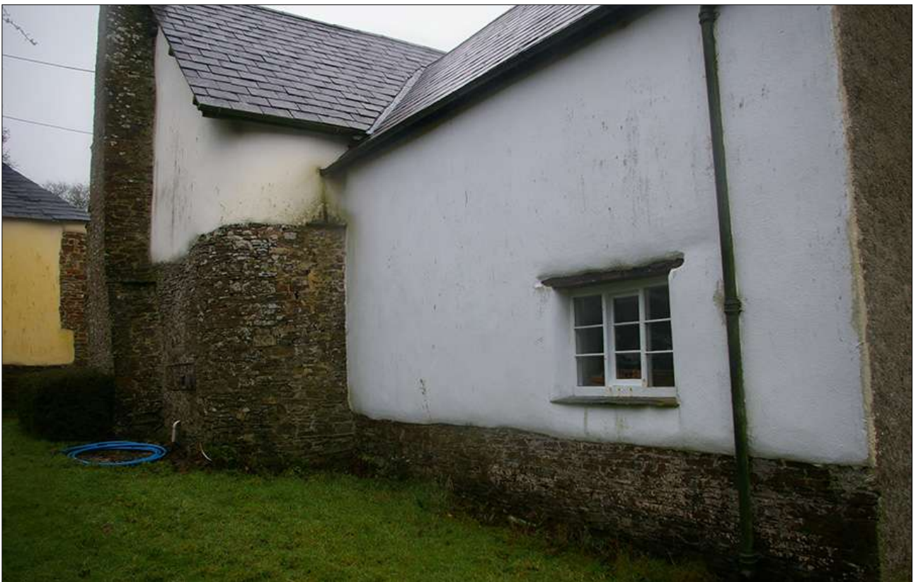
THE NORTH ELEVATION OF THE HOUSE AND CROSSWING, VIEWED FROM THE NORTH-WEST.
