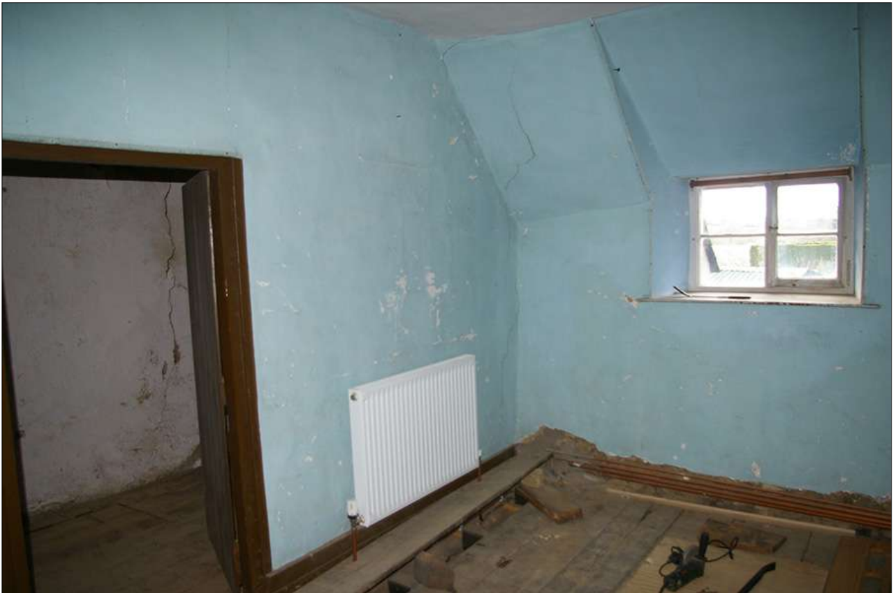
BEDROOM 4, SHOWING THE DOORWAY (D16) INTO THE APPLE STORE; VIEWED FROM THE NORTH-EAST.
