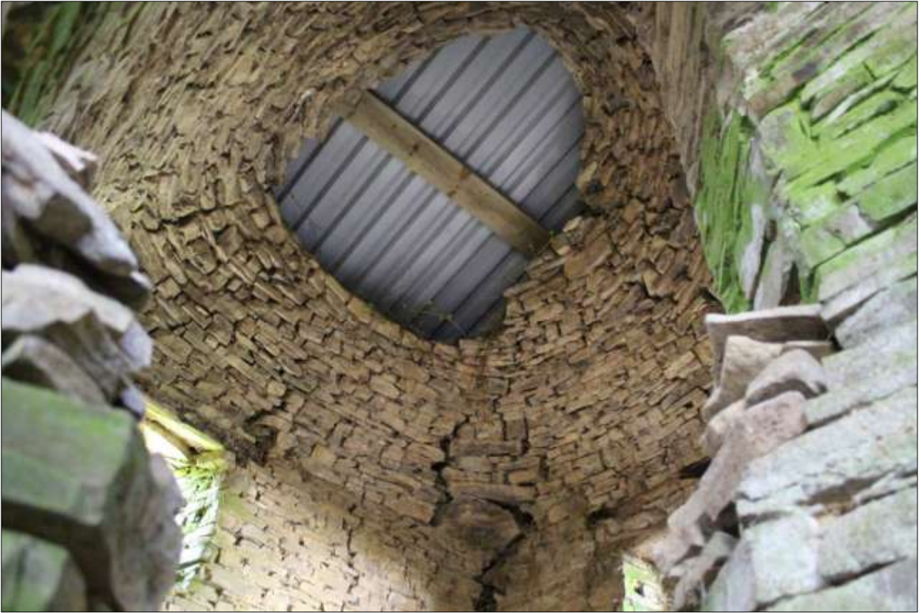
THE CORBELLED ROOF OF THE MALTING KILN, FROM THE ENTRANCE OF THE FLUE IN THE BACK OF THE FIREPLACE; VIEWED FROM THE SOUTH-EAST.
