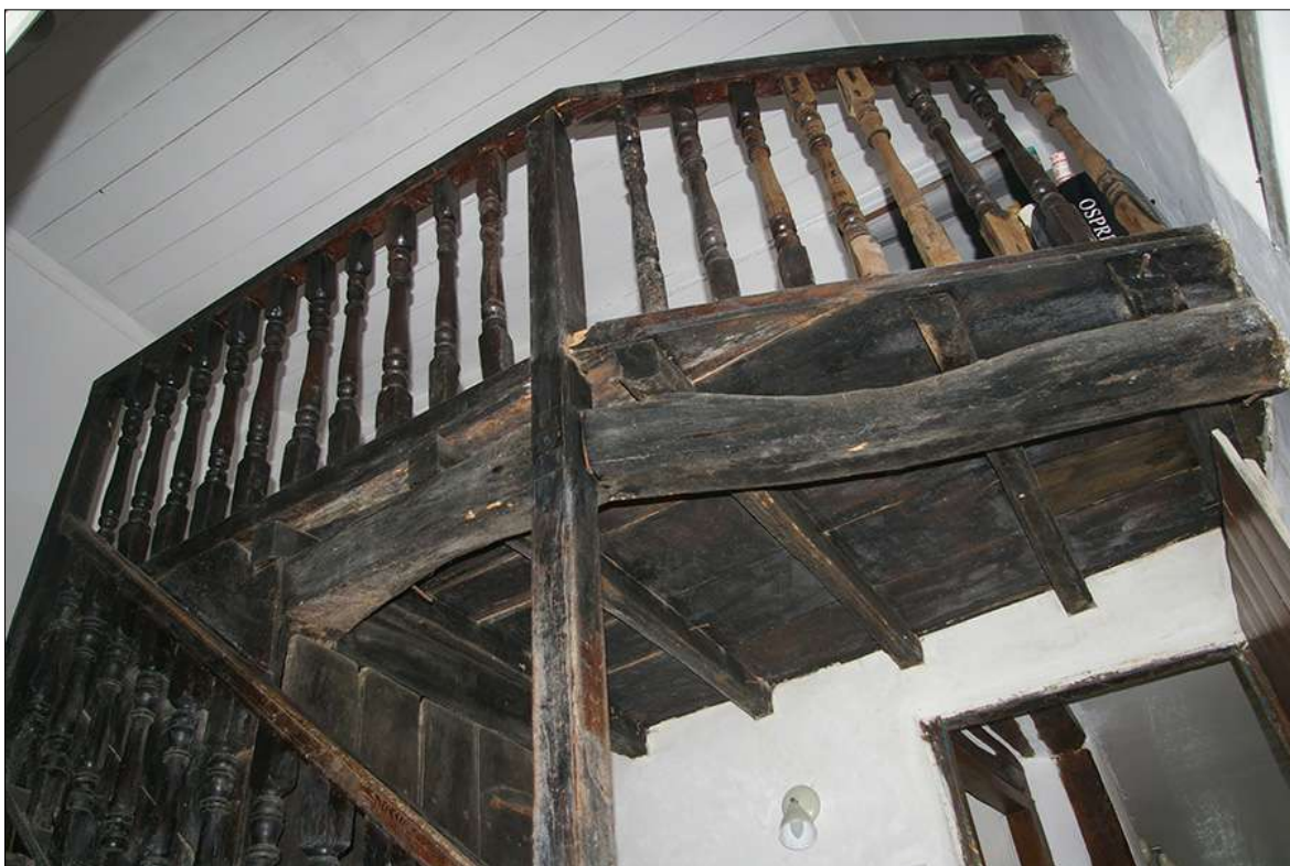
FIGURE 11: THE STAIRS IN THE STAIRHALL, VIEWED FROM BELOW AND TO THE SOUTH-WEST.
