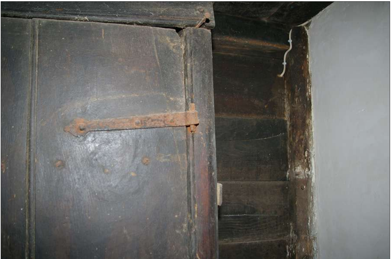
STAIRHALL, DETAIL OF THE HINGE OF THE UNDERSTAIR CUPBOARD DOOR; VIEWED FROM THE SOUTH.
