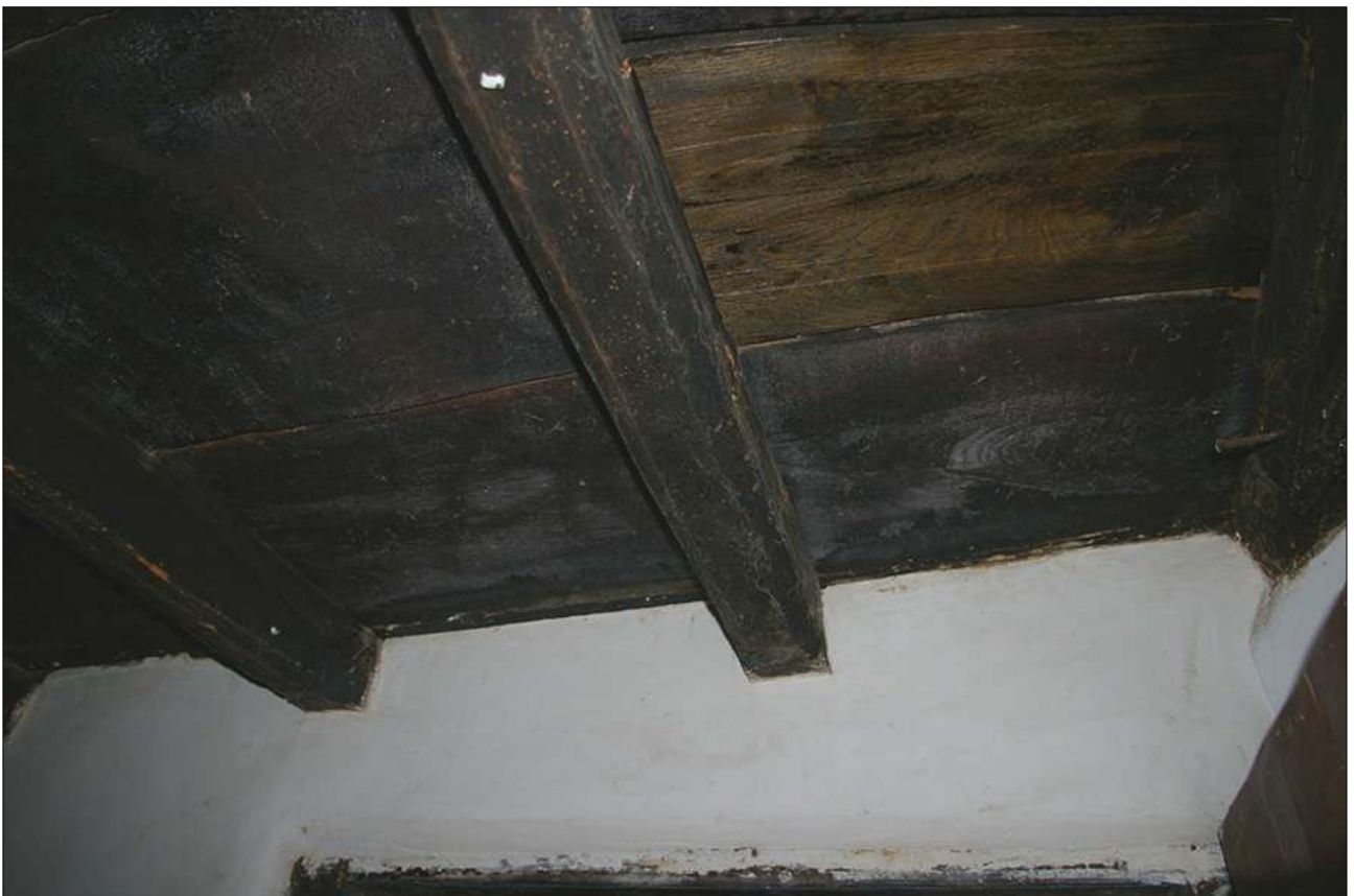
STAIRHALL, UNDERSIDE OF THE LANDING SHOWING JOISTS ABOVE D6; VIEWED FROM THE WEST.
