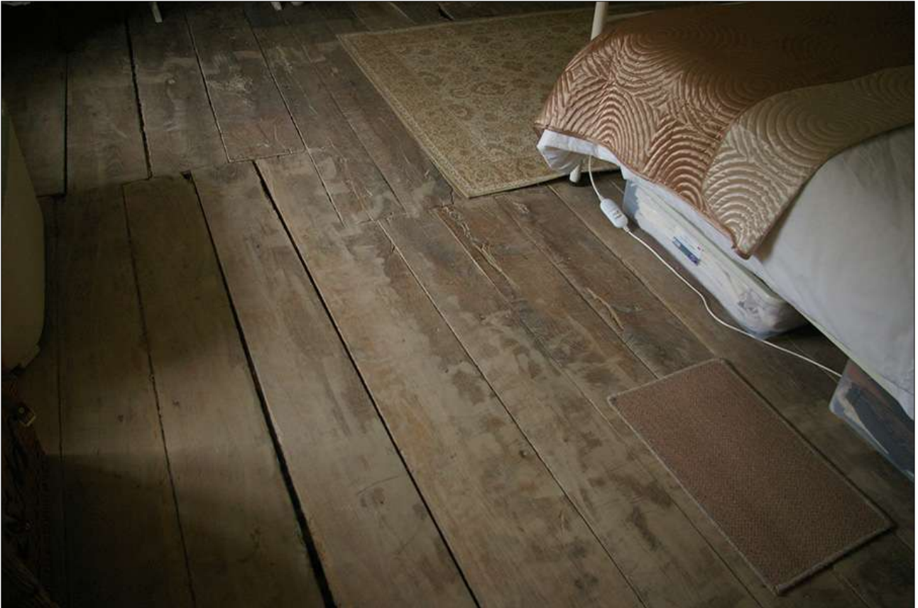
BEDROOM 1, DETAIL OF THE FLOORBOARDS NEXT TO THE WINDOW; VIEWED FROM THE NORTH.
