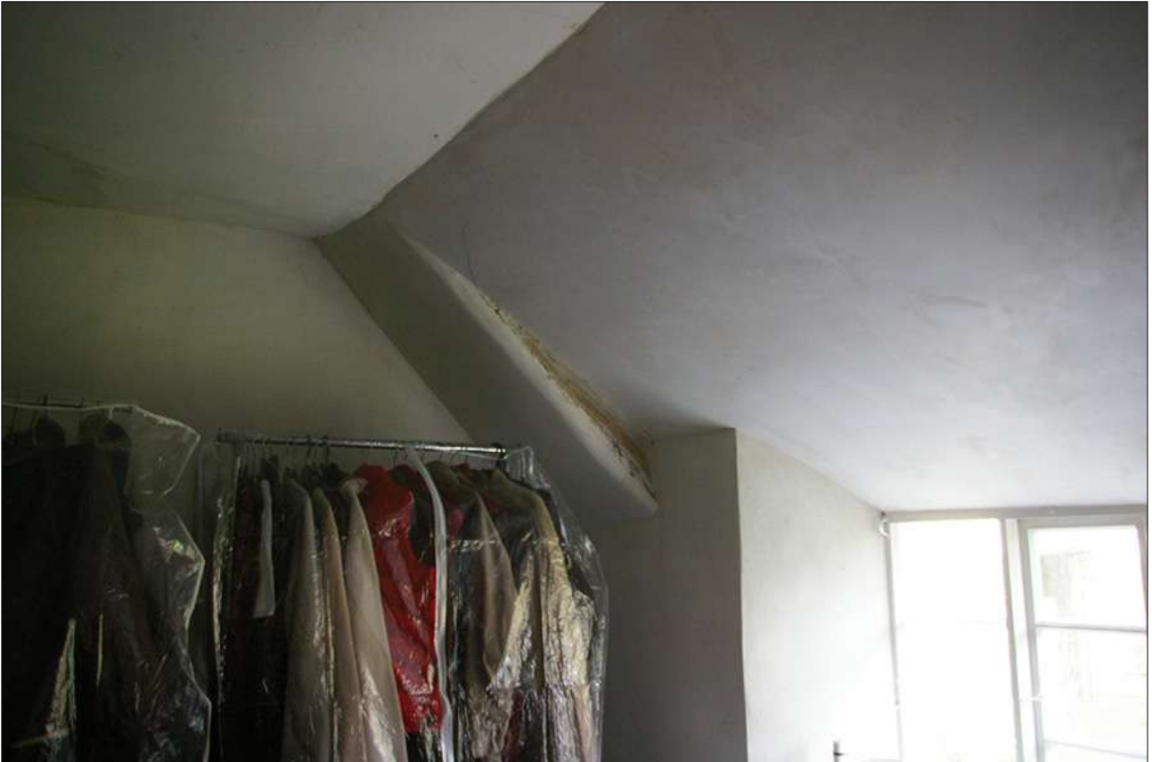
BEDROOM 3, SHOWING THE FOOT OF THE ROOF TRUSS NORTH OF THE W8; VIEWED FROM THE SOUTH-WEST.
