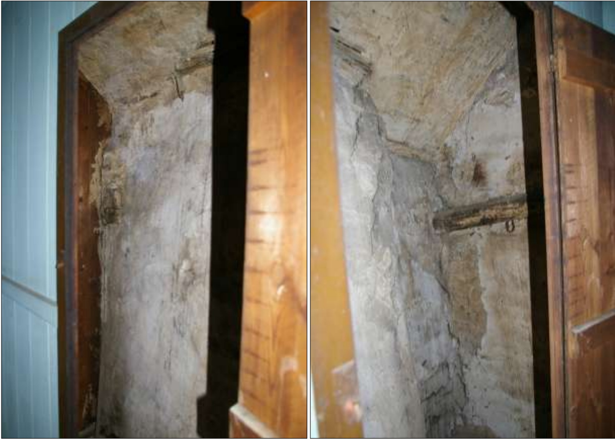
LEFT: THE NORTH SIDE OF THE AIRING CUPBOARD; VIEWED FROM THE SOUTH-WEST.
