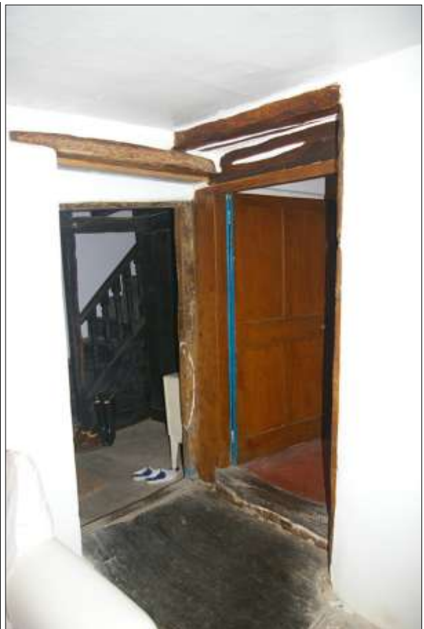
RIGHT: HALL, NORTH-WEST CORNER WITH DOORWAYS TO STAIRHALL (D6) AND PARLOUR (D7); VIEWED FROM THE SOUTH-EAST.
