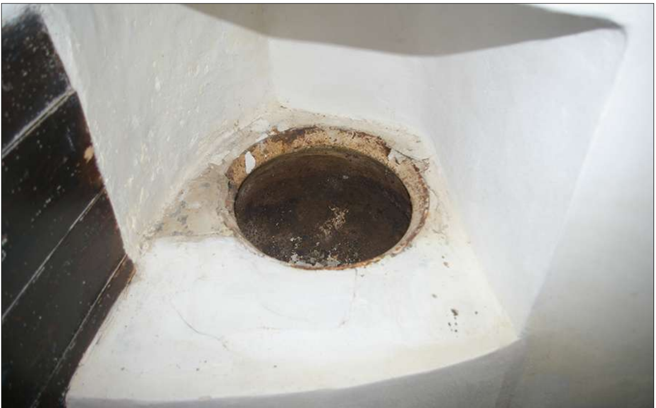
HALL, DETAIL OF THE BOILER/COPPER (S2); VIEWED FROM THE NORTH.
