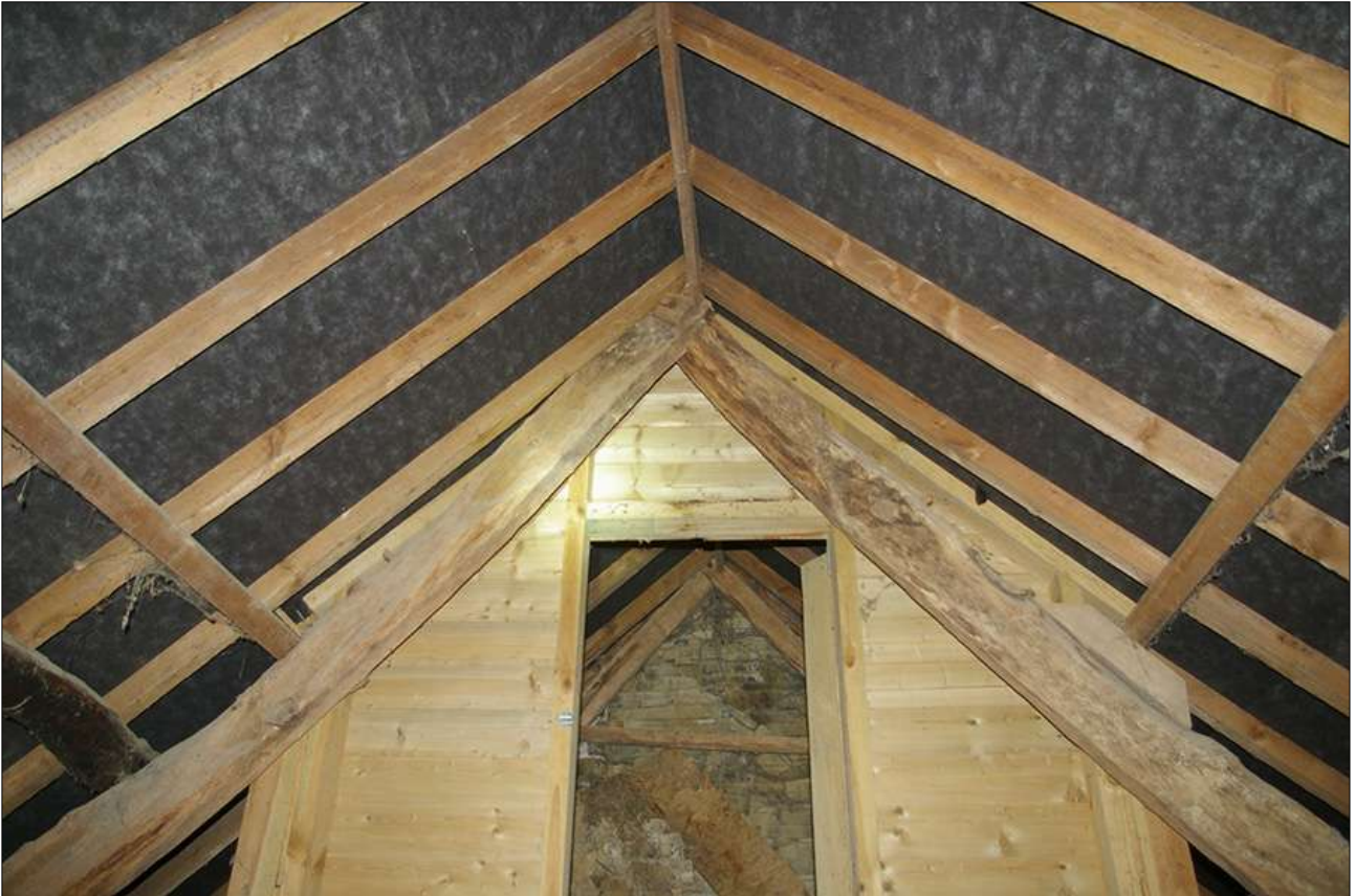
THE OWL-BOX AT THE NORTH END OF THE ROOFSPACE; VIEWED FROM THE SOUTH.
