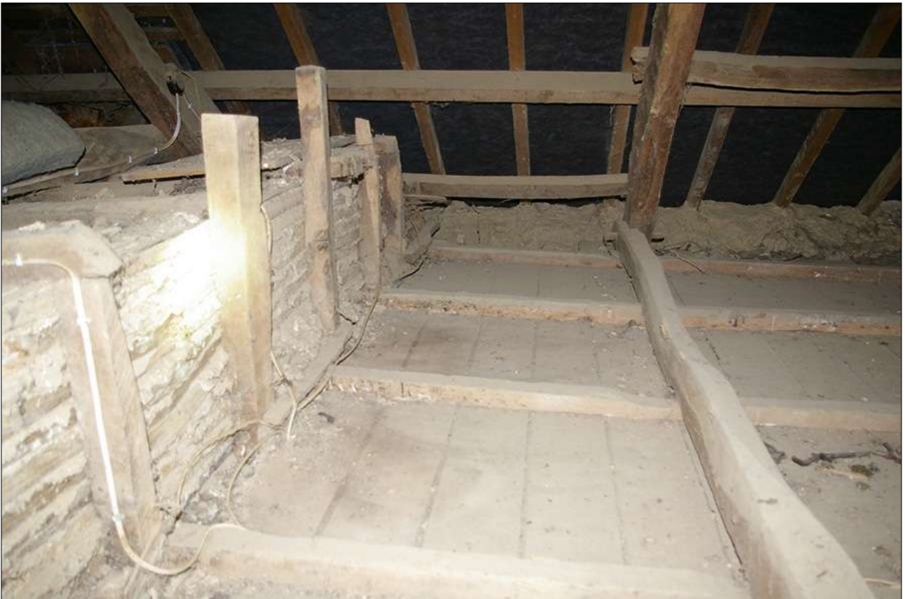
THE STEP HEIGHT IN THE CEILINGS BETWEEN THE APPLE STORE (RIGHT) AND BEDROOM 4 (LEFT); VIEWED FROM THE WEST.
