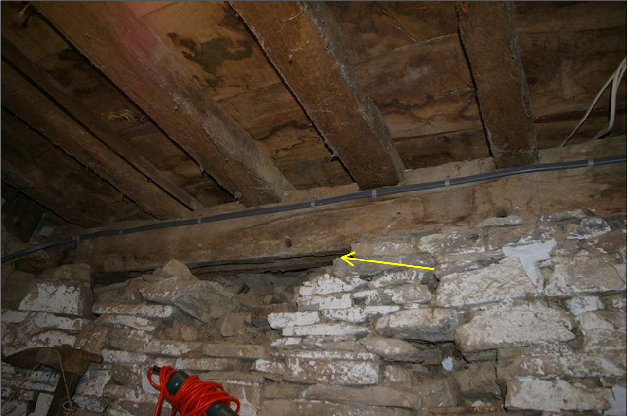
CROSS PASSAGE WEST END, NORTH WALL, SHOWING THE SLOTS IN THE UNDERSIDE OF THE BEAM (INDICATED); VIEWED FROM THE SOUTH.
