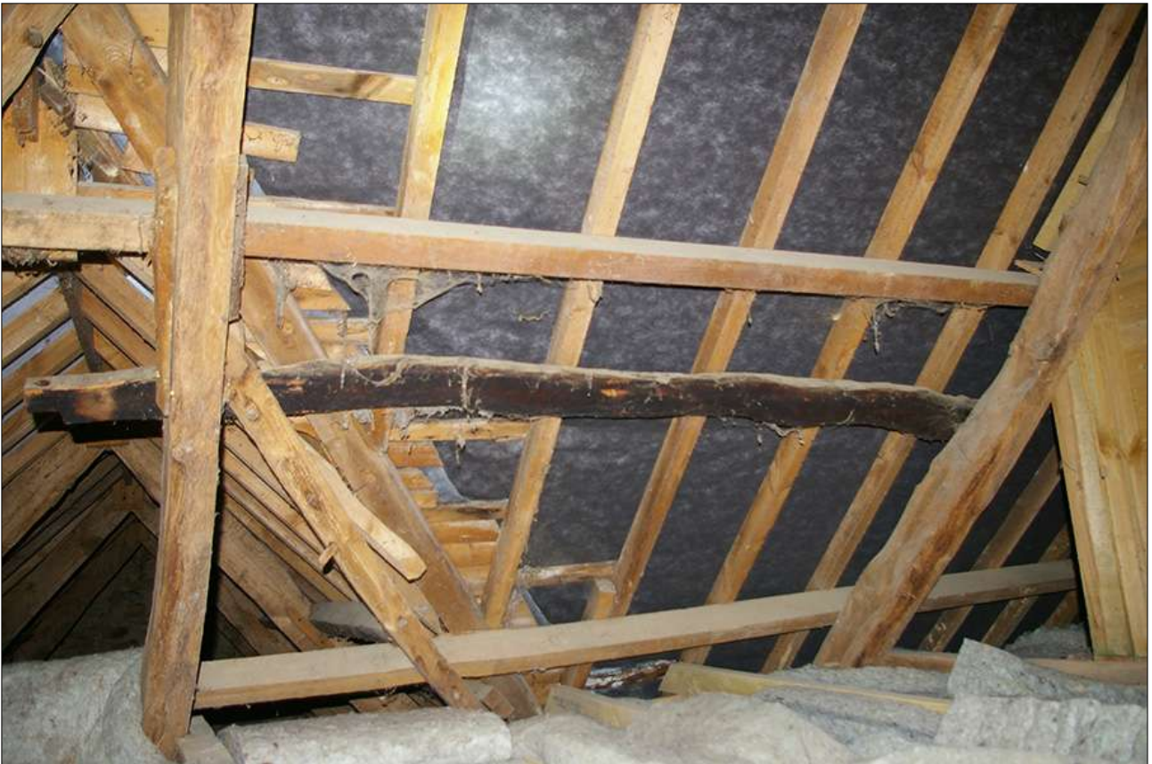
THE ROOF ABOVE BEDROOM 2, WEST PITCH, AT THE JUNCTION WITH THE CROSSWING, SHOWING THE SINGLE SMOKE-BLACKENED REUSED RAFTER; VIEWED FROM THE EAST.
