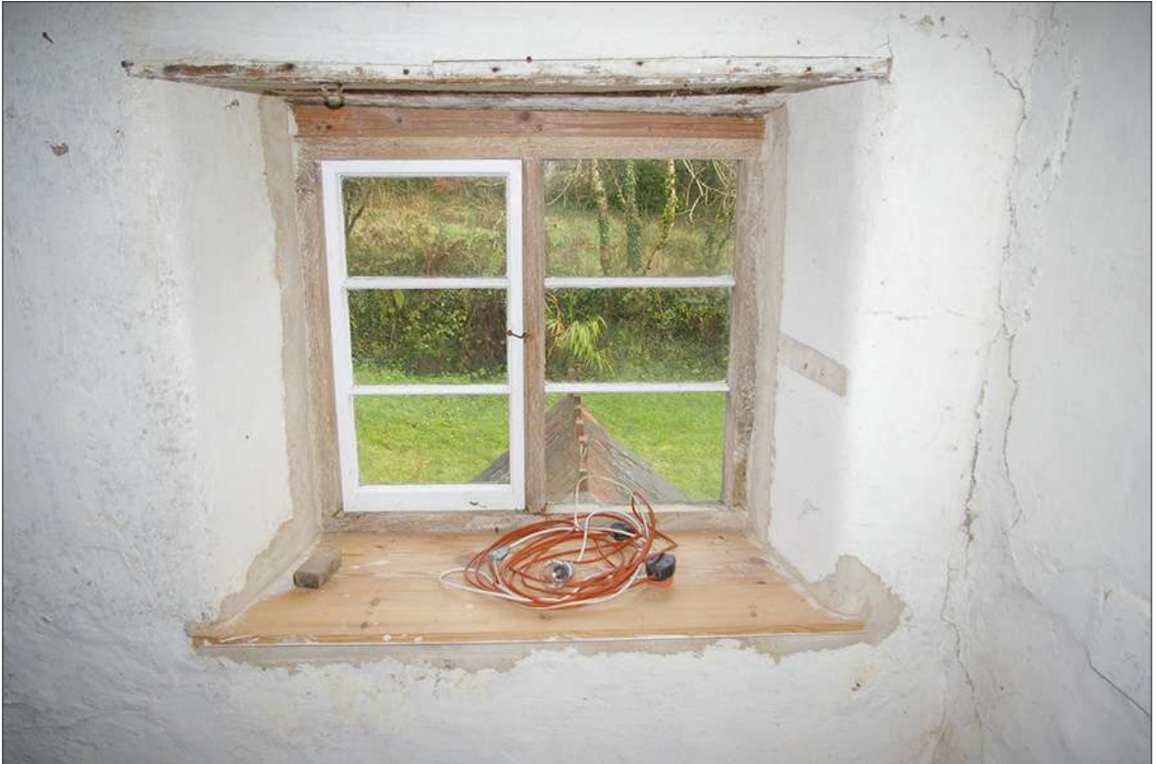
APPLE STORE, DETAIL OF THE WEST WINDOW (W7); VIEWED FROM THE EAST.
