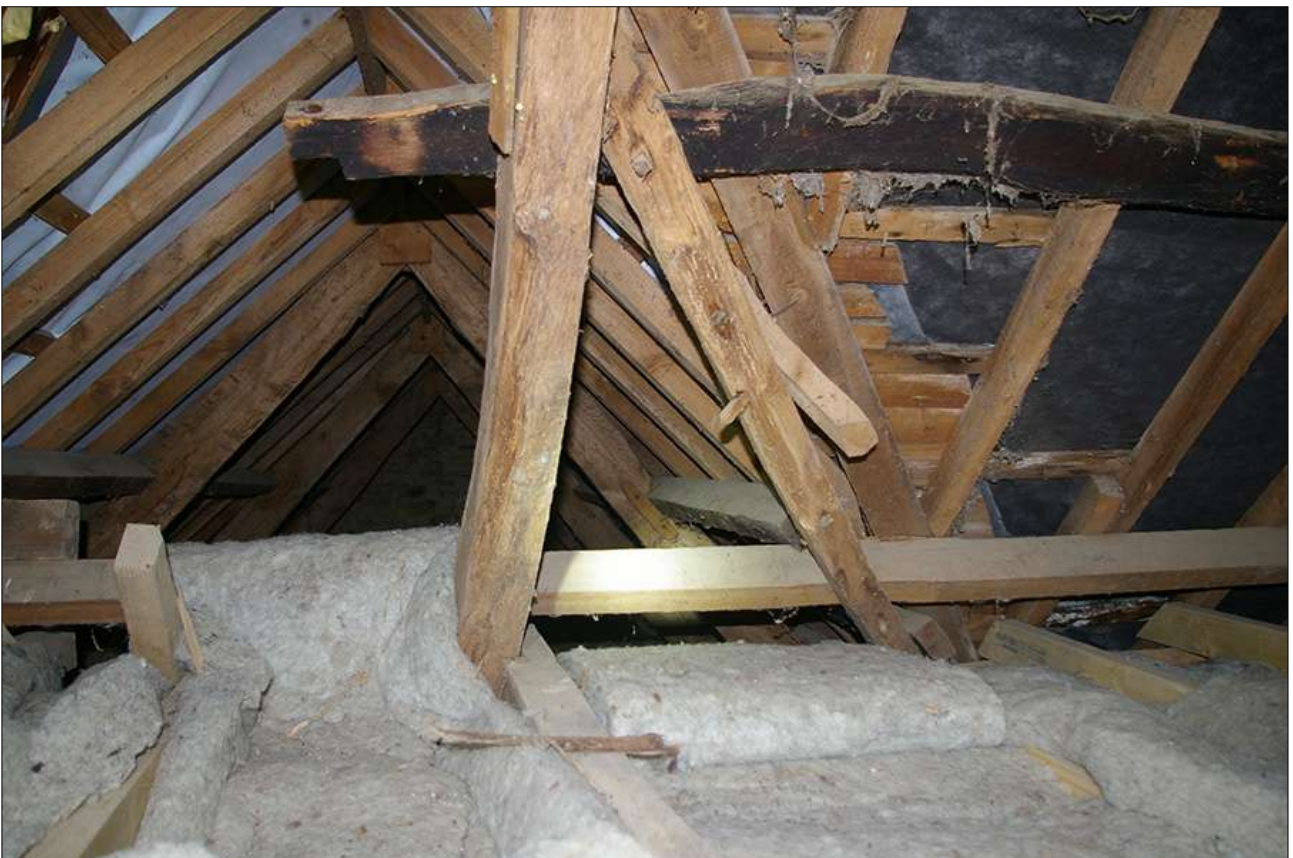
AS ABOVE, DETAIL OF THE SMOKE-BLACKENED PURLIN.
