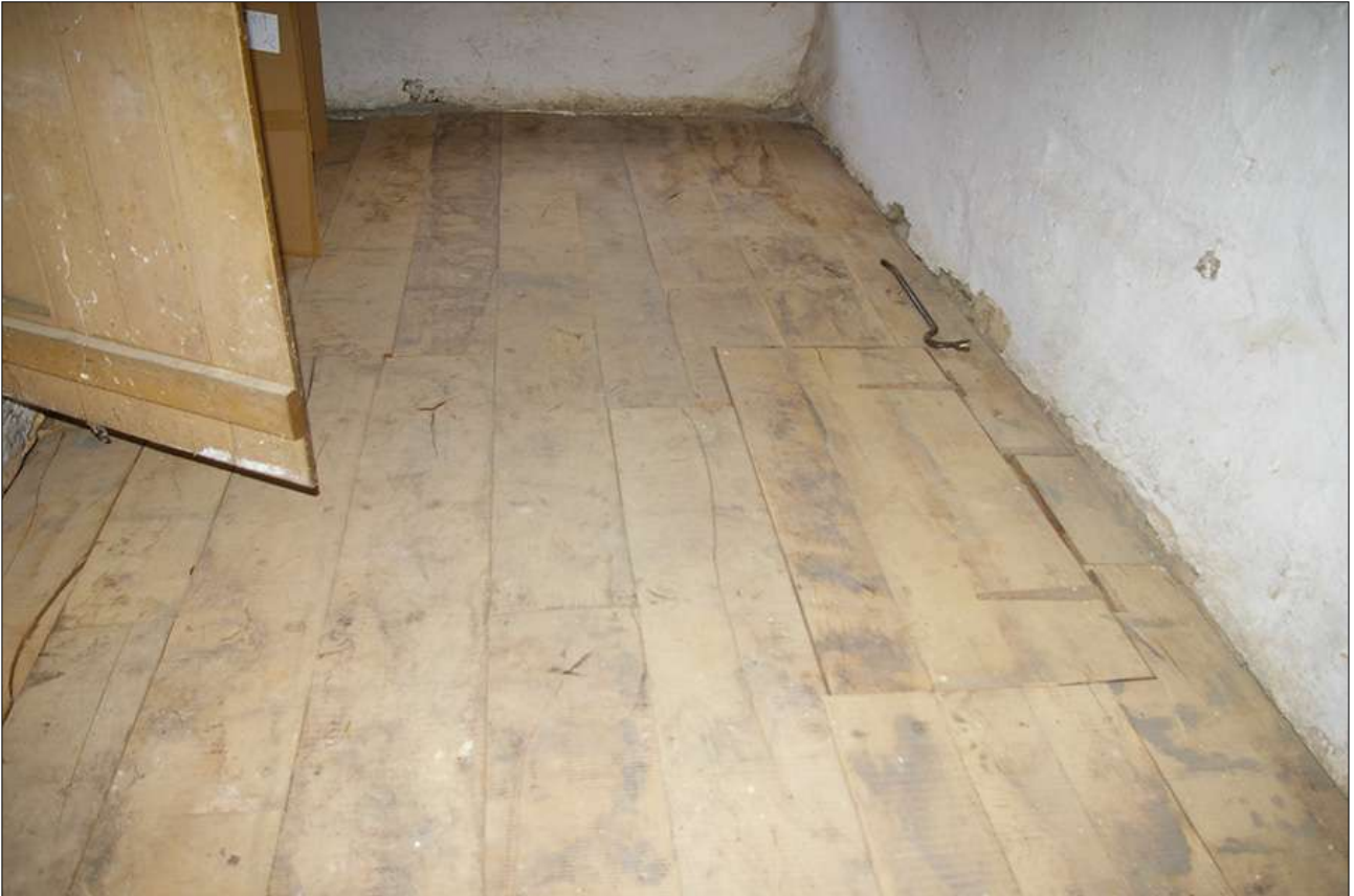
APPLE STORE, DETAIL OF THE NEW OAK FLOORBOARDS AND HATCH INTO THE PASSAGE; VIEWED FROM THE SOUTH.
