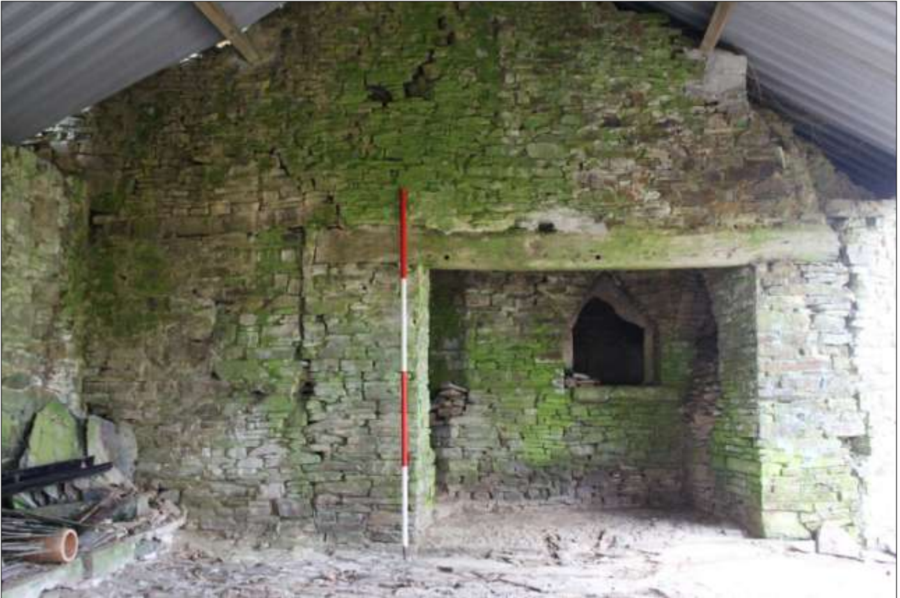
THE INTERNAL WALL OF THE BAKEHOUSE; VIEWED FROM THE SOUTH-WEST (SCALE 2M).
