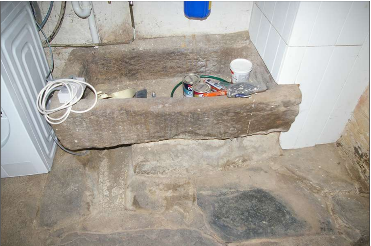
PUMP ROOM, DETAIL OF THE GRANITE TROUGH; VIEWED FROM THE EAST.
