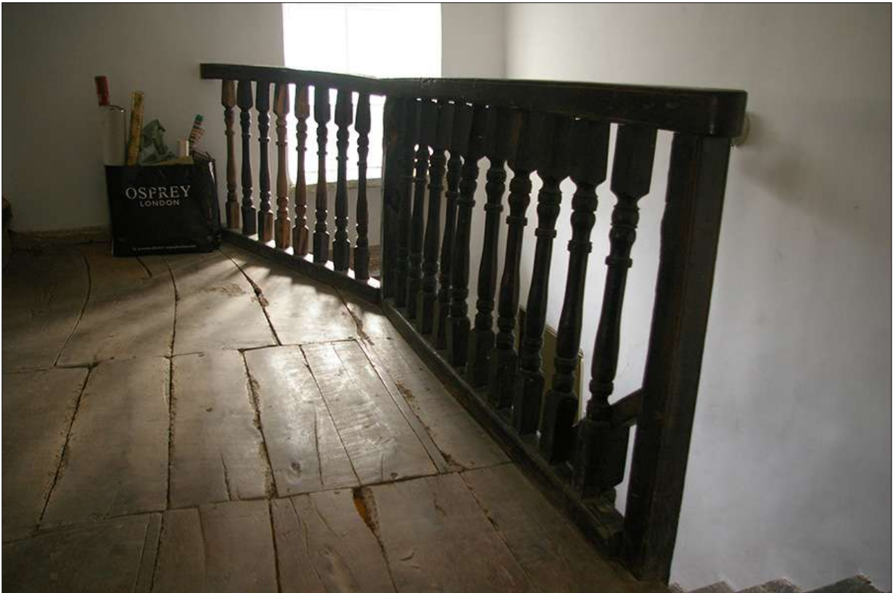
STAIRHALL FF, VIEW OF THE LANDING FLOOR AND STAIR RAIL; VIEWED FROM THE NORTH.
