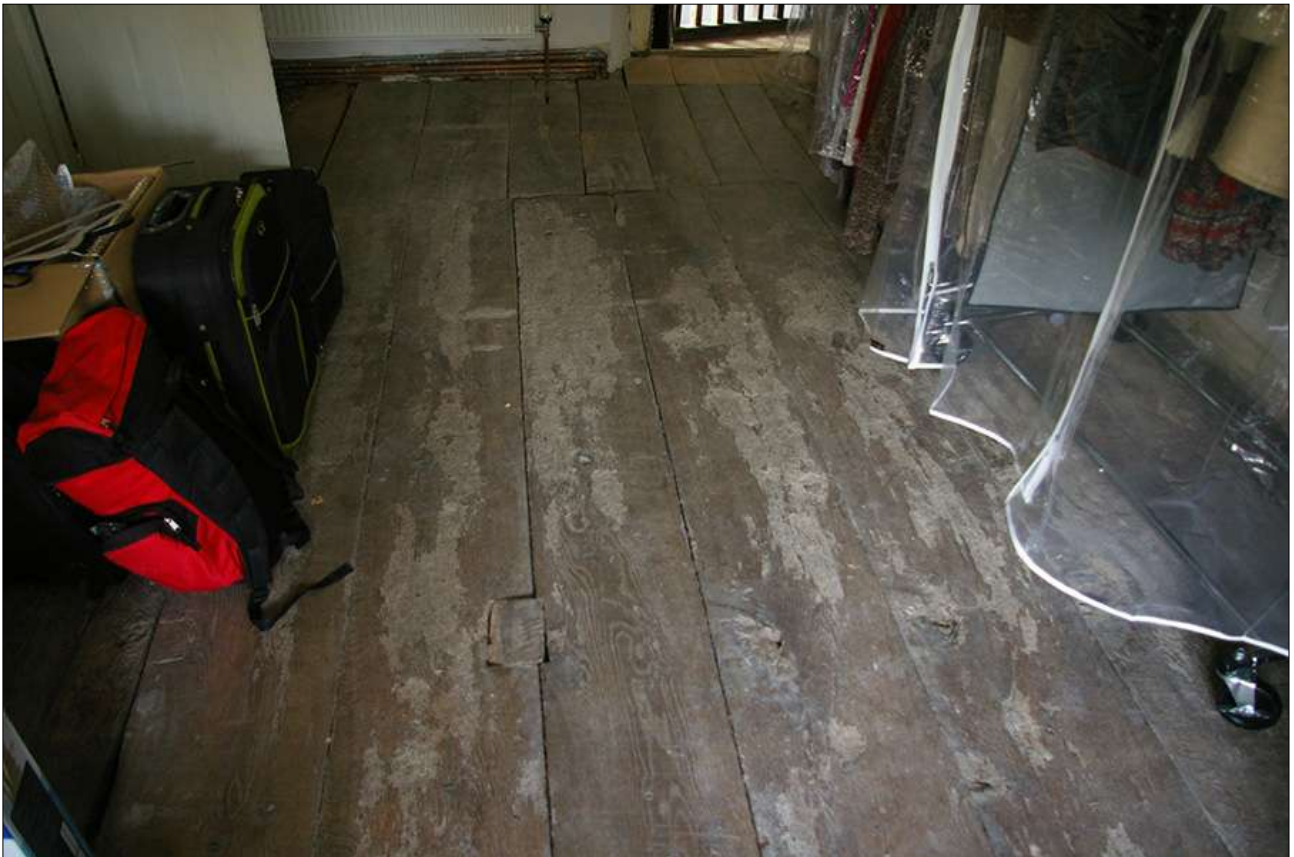
BEDROOM 3, THE FLOORBOARDS; VIEWED FROM THE EAST.
