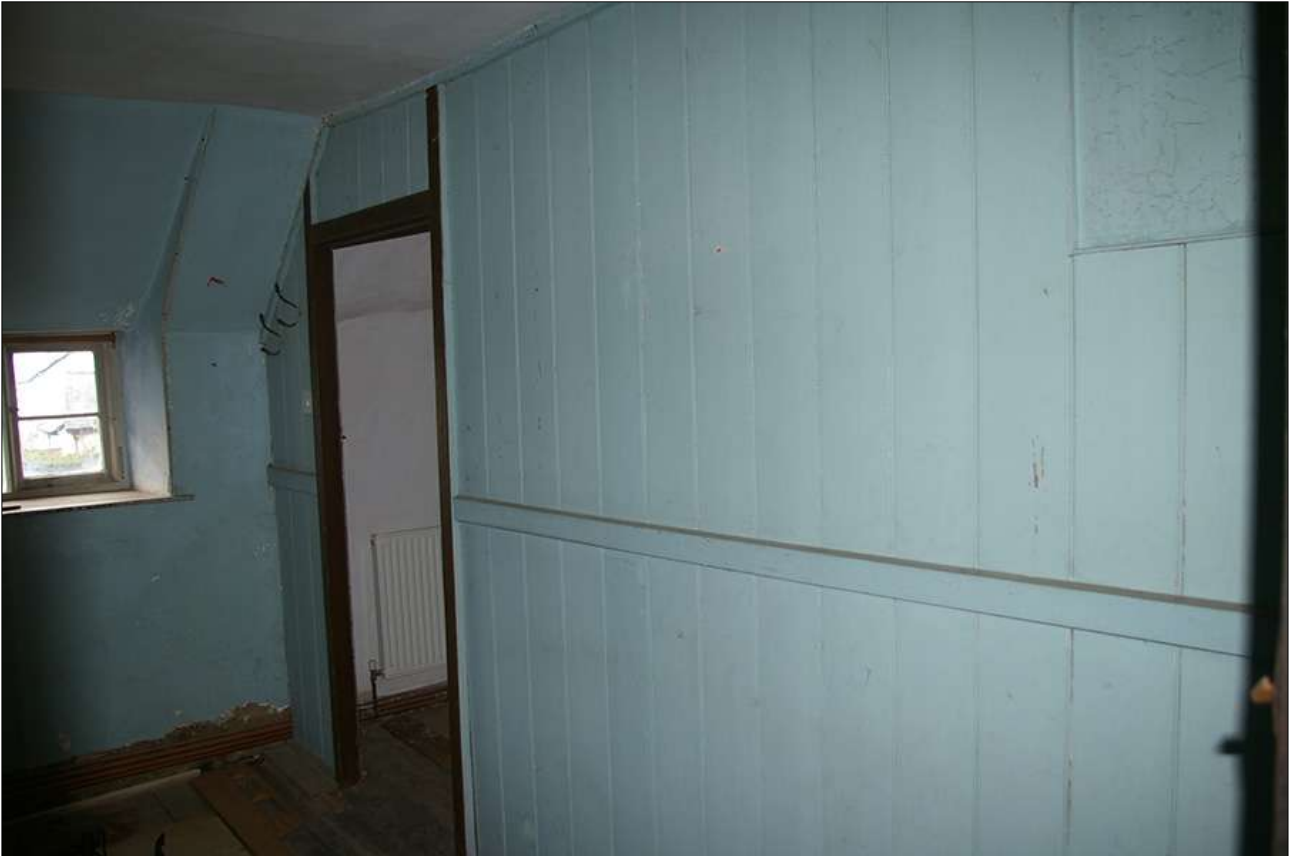
BEDROOM 4, SHOWING THE NORTH PARTITION WALL WITH BEDROOM 3 AND DOORWAY (D14); VIEWED FROM THE EAST-SOUTH-EAST.
