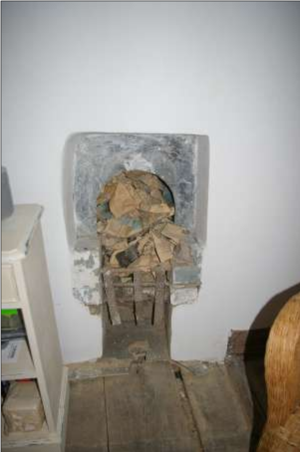
BEDROOM 1, DETAIL OF THE FORCED GRATE IN THE NORTH WALL; VIEWED FROM THE SOUTH.
