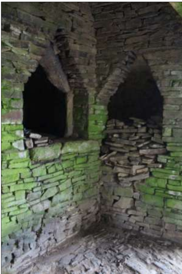
THE OVENS IN THE BACK OF THE FIREPLACE; VIEWED FROM THE WEST-SOUTH-WEST.
