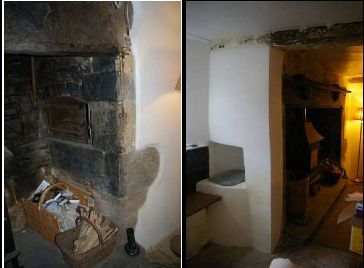
LEFT: HALL, FP1, SHOWING THE DRESSED FREESTONE AND BREAD OVEN; VIEWED FROM THE NORTH-WEST.
