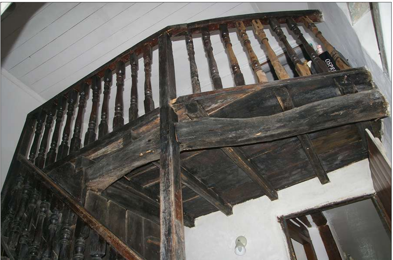
STAIRHALL, THE STAIRS AND SPINDLES ON THE FIRST FLOOR; VIEWED FROM THE WEST.
