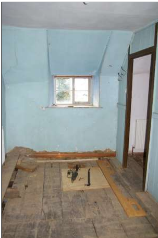
BEDROOM 4, SHOWING THE WESTERN END OF THE ROOM AND WINDOW (W12); VIEWED FROM THE EAST.
