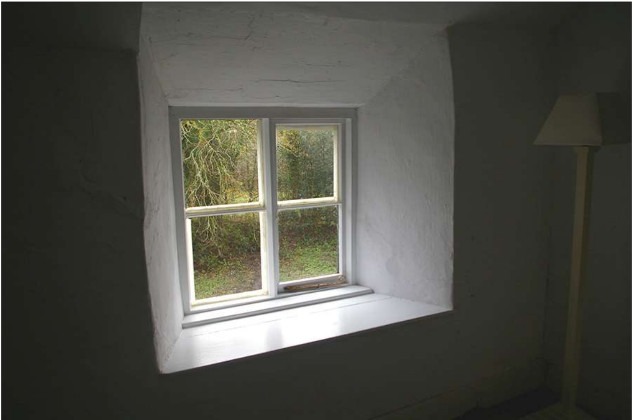
BEDROOM 1, THE WINDOW (W10) IN THE SOUTH WALL; VIEWED FROM THE NORTH-EAST.
