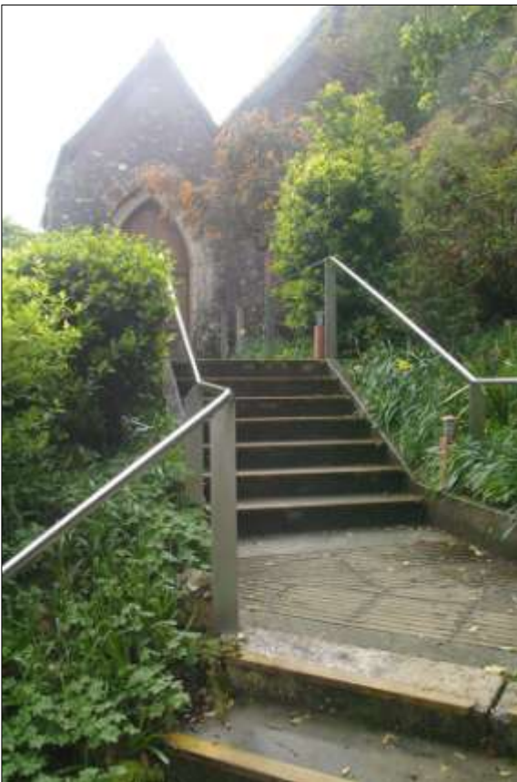
THE UNSYMPHATICALLY-RESTORED STEPS LEADING TO ST ANDREW'S CHURCH; VIEWED FROM THE NORTH-WEST.
