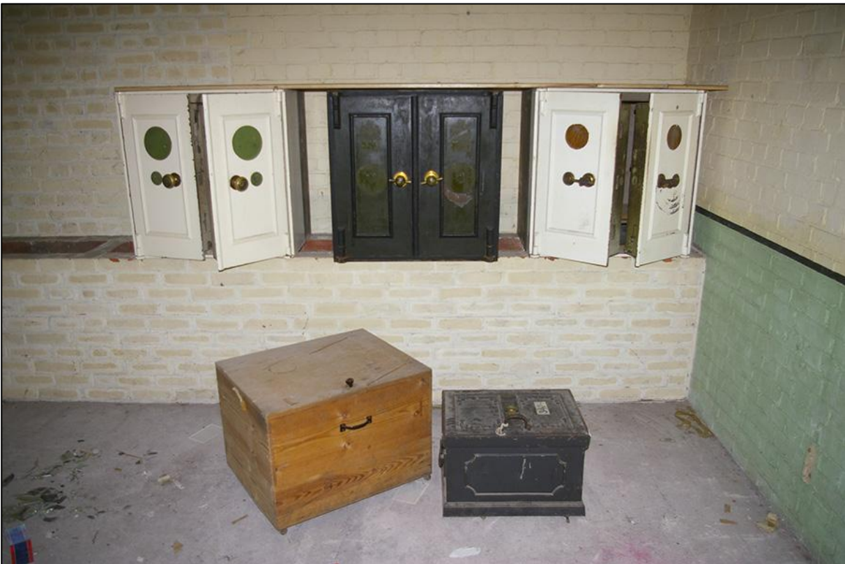
SAFES IN BASEMENT OF OFFICE BLOCK (BUILDING 13), SHOWING PROBABLE ORIGINAL PAINT WORK.
