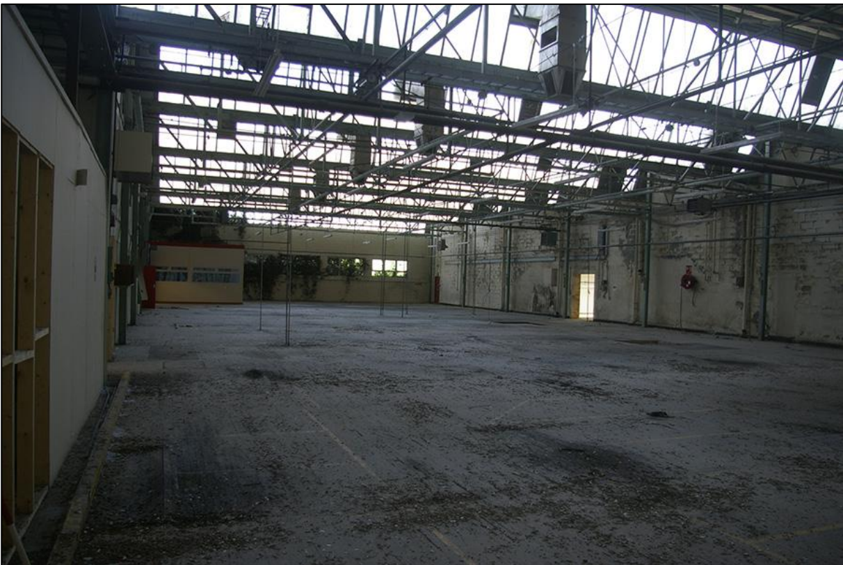
SOUTH-EAST END OF BUILDING 11, WHERE THE ORIGINAL ROAD BETWEEN THE WAREHOUSES AND MAIN FACTORY WAS INFILLED WITH THIS AND OTHER STRUCTURES; VIEWED FROM THE WEST-SOUTH-WEST.
