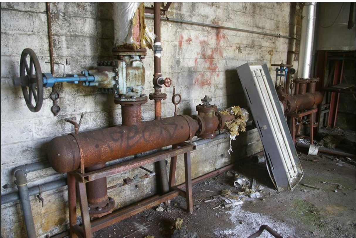
PLANT WITHIN SOUTH-WEST SIDE OF BUILDING 8 (PLANT ROOM); VIEWED FROM THE SOUTH.
