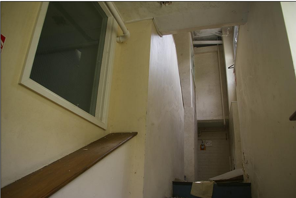
ORIGINAL DEFENSIBLE/BLAST DEFENSE, CENTRAL STAIRED ENTRANCE TO OFFICE BLOCK (BUILDING 13); VIEWED FROM THE NORTH-EAST.
