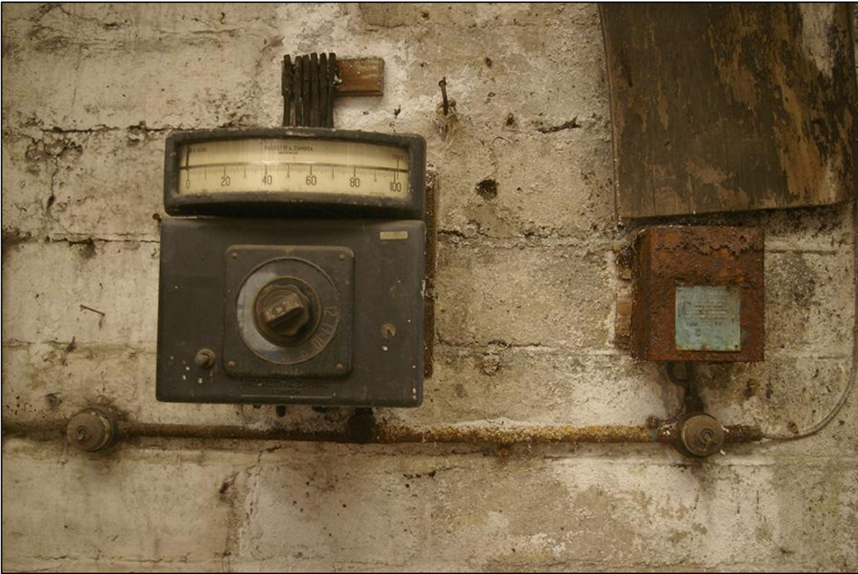
MACHINERY ON SOUTH-EAST ELEVATION WITHIN NORTH-EAST SIDE OF BUILDING 8 (PLANT ROOM); VIEWED FROM THE NORTH-WEST.
