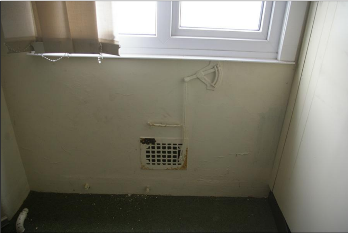
VENT IN FIRST FLOOR OFFICE OF OFFICES (BUILDING 13); VIEWED FROM THE NORTH-WEST.
