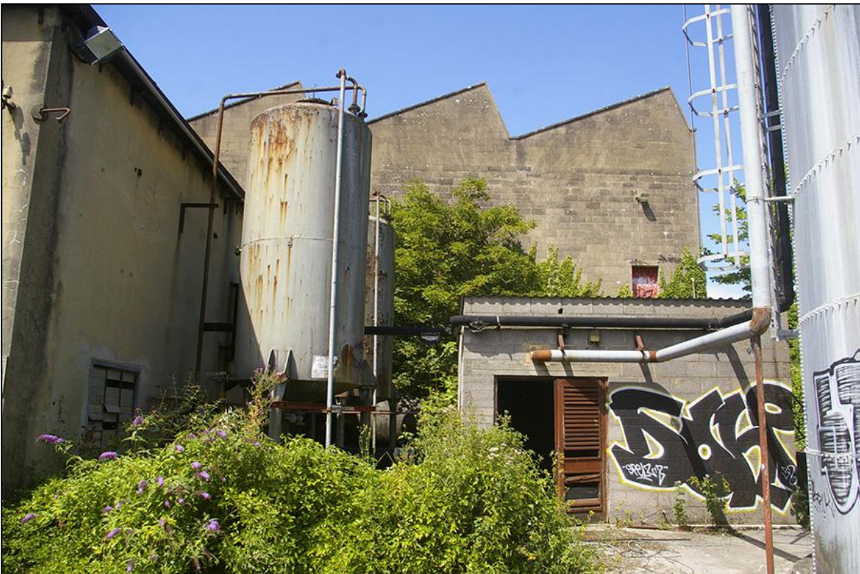
GENERATOR SHED (BUILDING 10), EDGE OF TANK AND SOUTH-EAST ELEVATION OF BUILDING 11; VIEWED FROM THE SOUTH-EAST.
