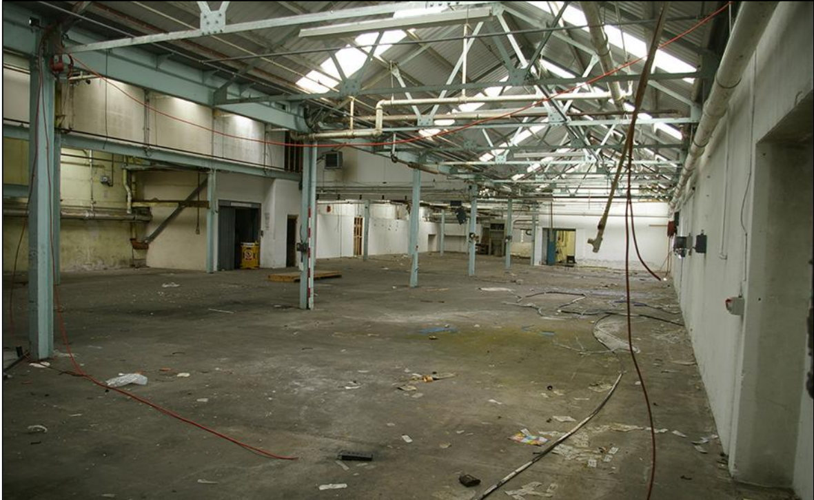
FIGURE 3: INTERIOR OF INFILL BEHIND MAIN FACTORY (BUILDING 1A); VIEWED FROM THE SOUTH.
