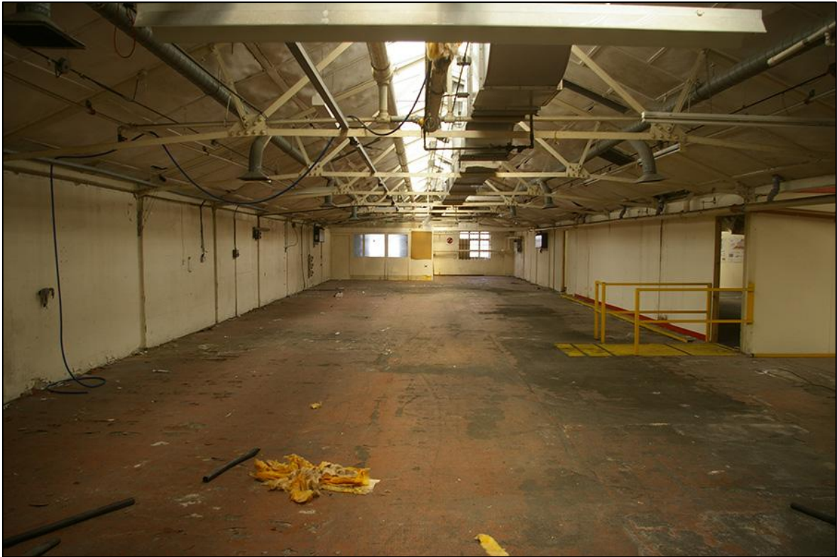
FIGURE 9: INTERIOR OF ONE OF THE BAYS WITHIN THE SINGLE STOREY BUILDING 11; VIEWED FROM THE SOUTH-WEST.
