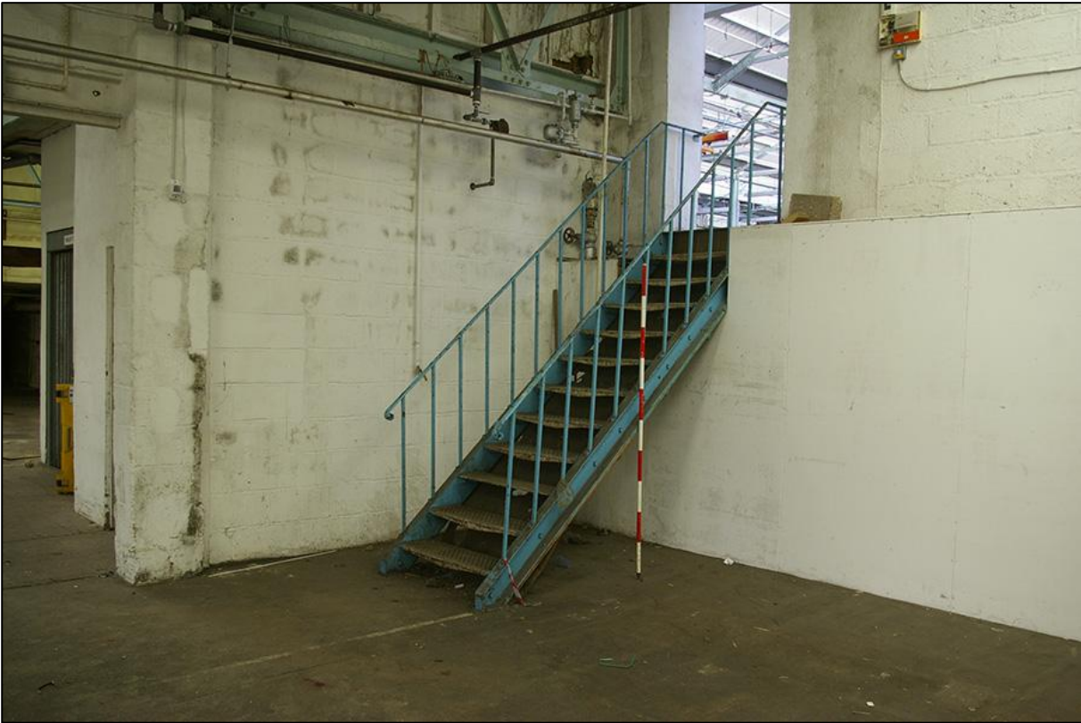
WROUGHT IRON STAIRCASE IN NORTH-EAST HALF OF BUILDING 1A, LEADING TO THE MAIN FACTORY (BUILDING 1); VIEWED FROM THE EAST (2M SCALE).
