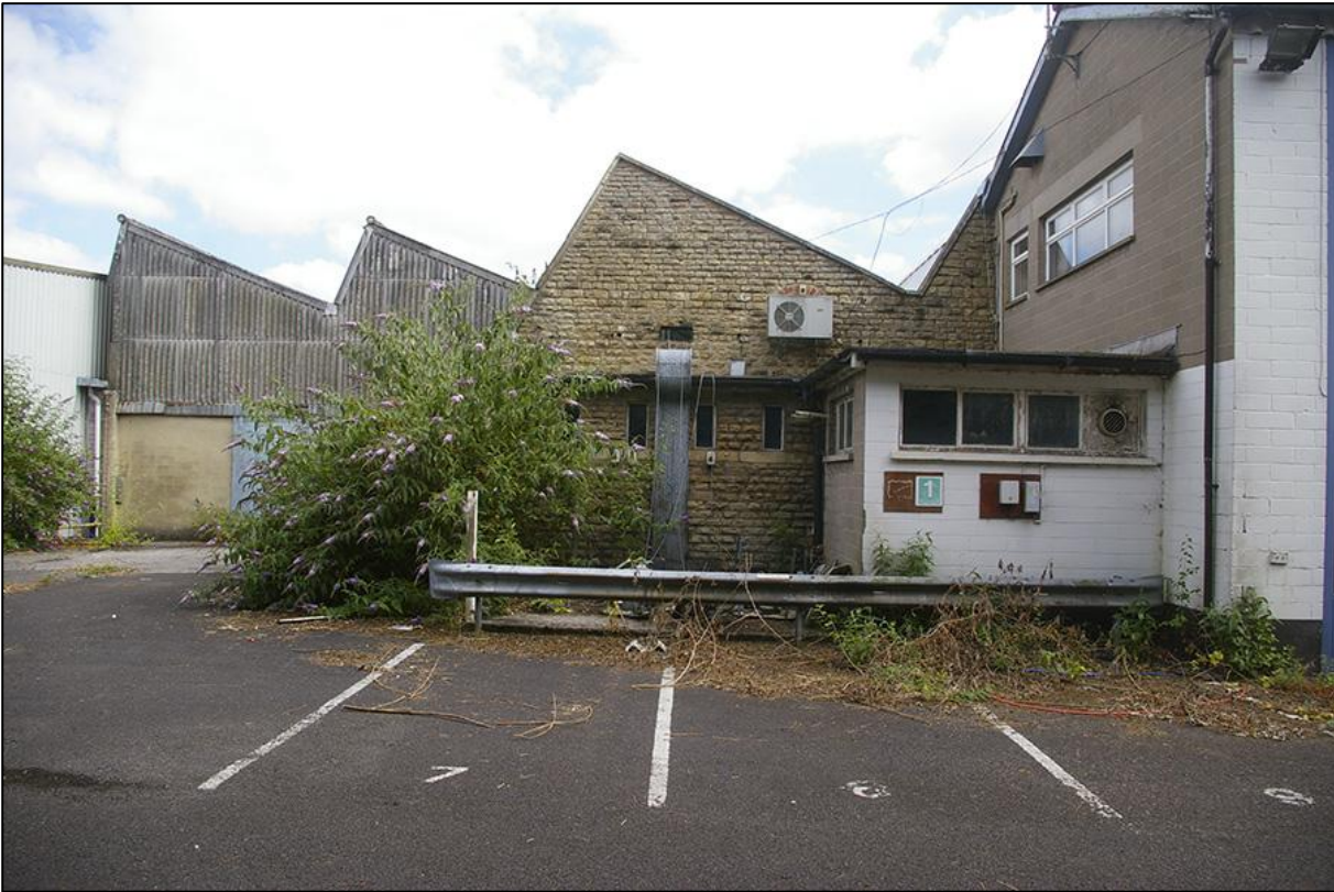
ELEVATION OF MAIN FACTORY (BUILDING 1) NORTH-EAST OF OFFICE BLOCK (BUILDING 13); VIEWED FROM THE NORTH-WEST.
