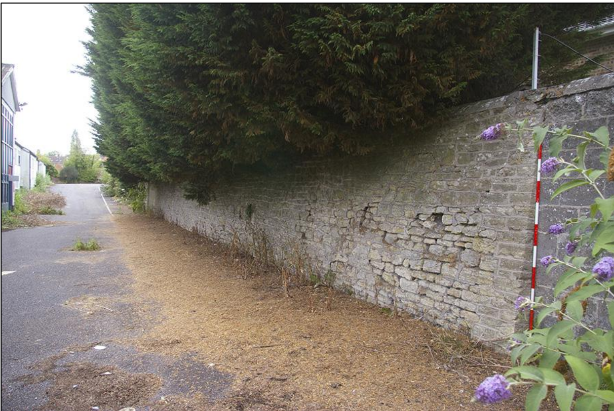
BOUNDARY WALL OPPOSITE ENTRANCE TO OFFICE BLOCK (BUILDING 13); VIEWED FROM THE EAST-NORTH-EAST (2M SCALE).
