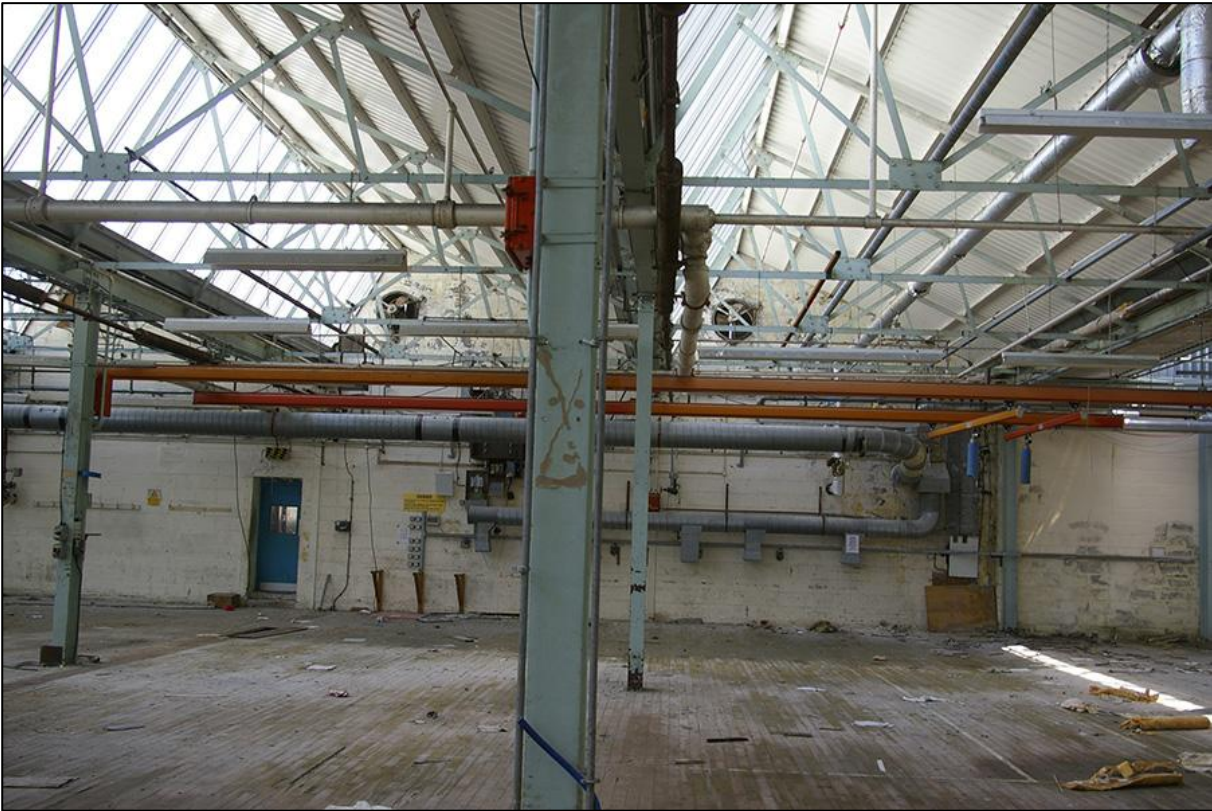
MAIN FACTORY (BUILDING 1), SHOWING BAY STYLE ROOFING AND AIR DUCTS/VENTS IN BRICK ROUNDELS; VIEWED FROM THE NORTH-WEST.
