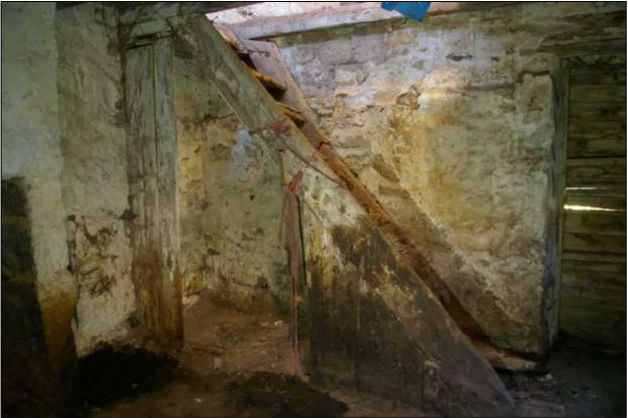
126. B3 GF INTERIOR, CLEARED OF RUBBISH, DETAIL OF THE STAIR; VIEWED FROM THE NORTH.
