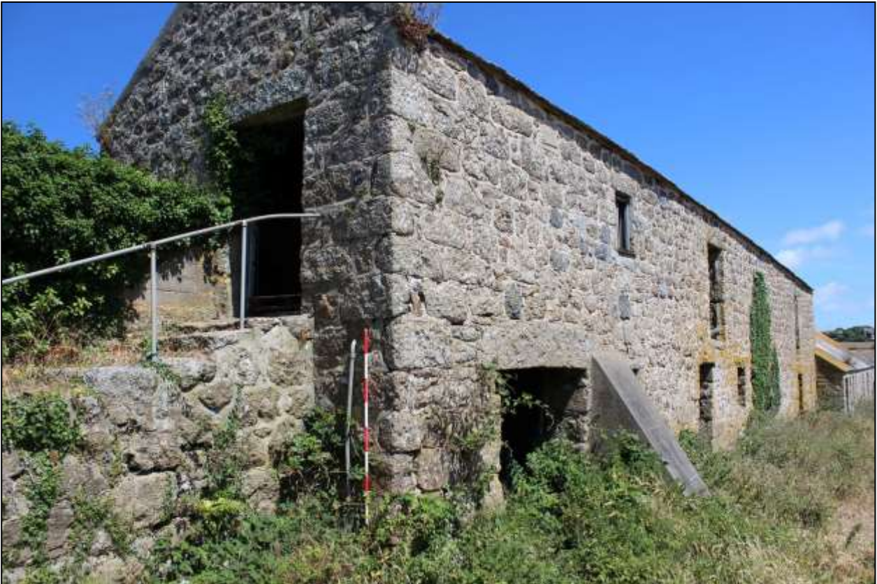
62. B9, SOUTH-WEST GABLE AND SOUTH-EAST ELEVATIONS; VIEWED FROM THE SOUTH (SCALE 2M).
