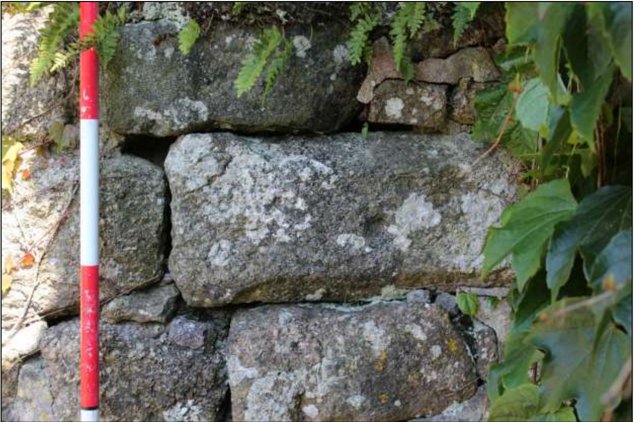
14. B4, SOUTH-EAST ELEVATION, DETAIL OF REUSED STONE IN WALL NEXT TO GD1; VIEWED FROM THE SOUTH (SCALE 2M).
