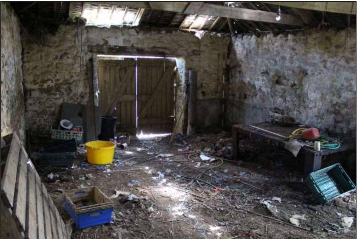
161. B7 INTERIOR, THE SOUTH-EAST WALL WITH GD4; VIEWED FROM THE NORTH-WEST (SCALE 2M).
