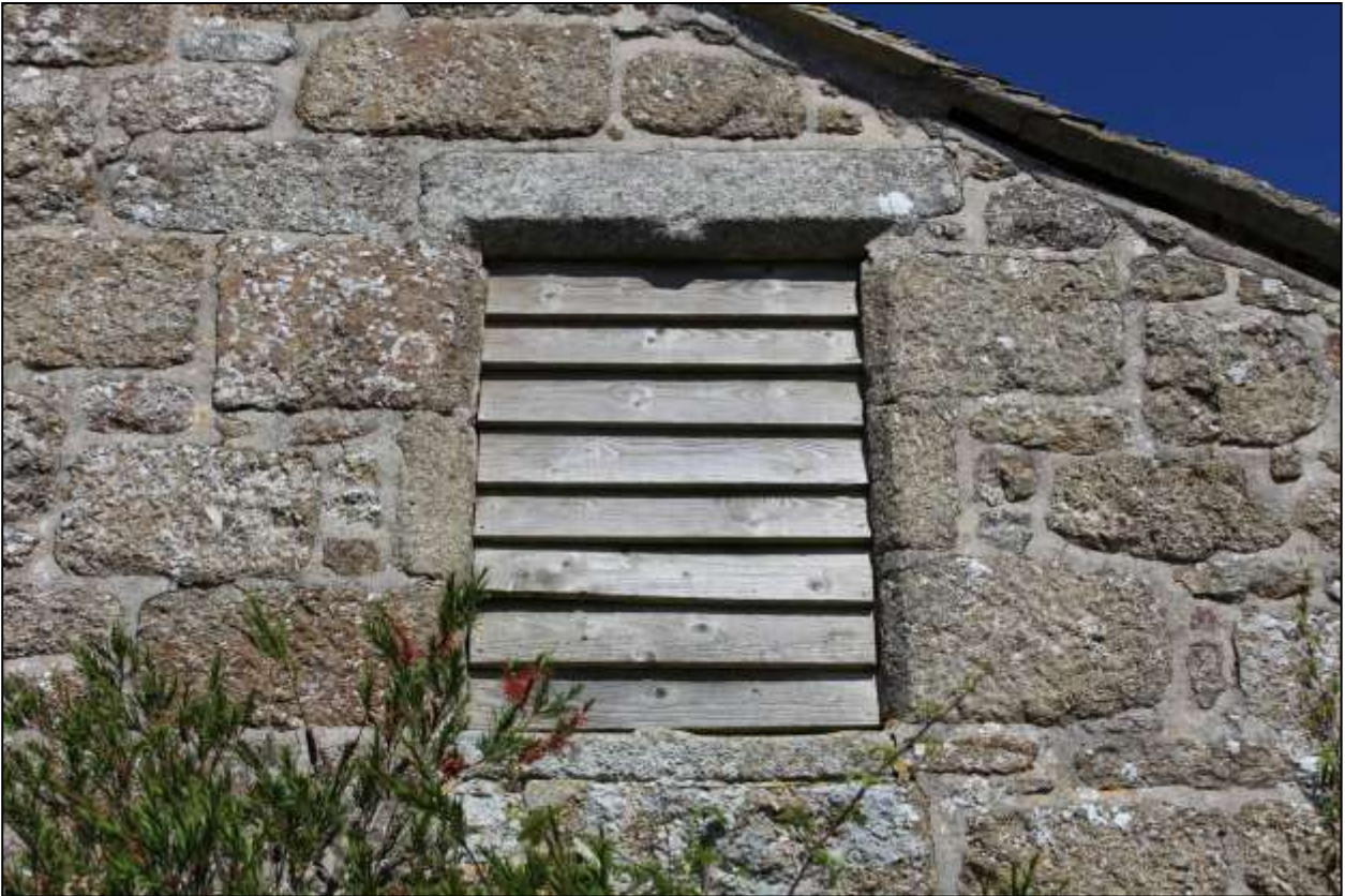
9. B3, FW2 IN THE SOUTH-EAST ELEVATION; VIEWED FROM THE SOUTH-EAST (SCALE 2M).
