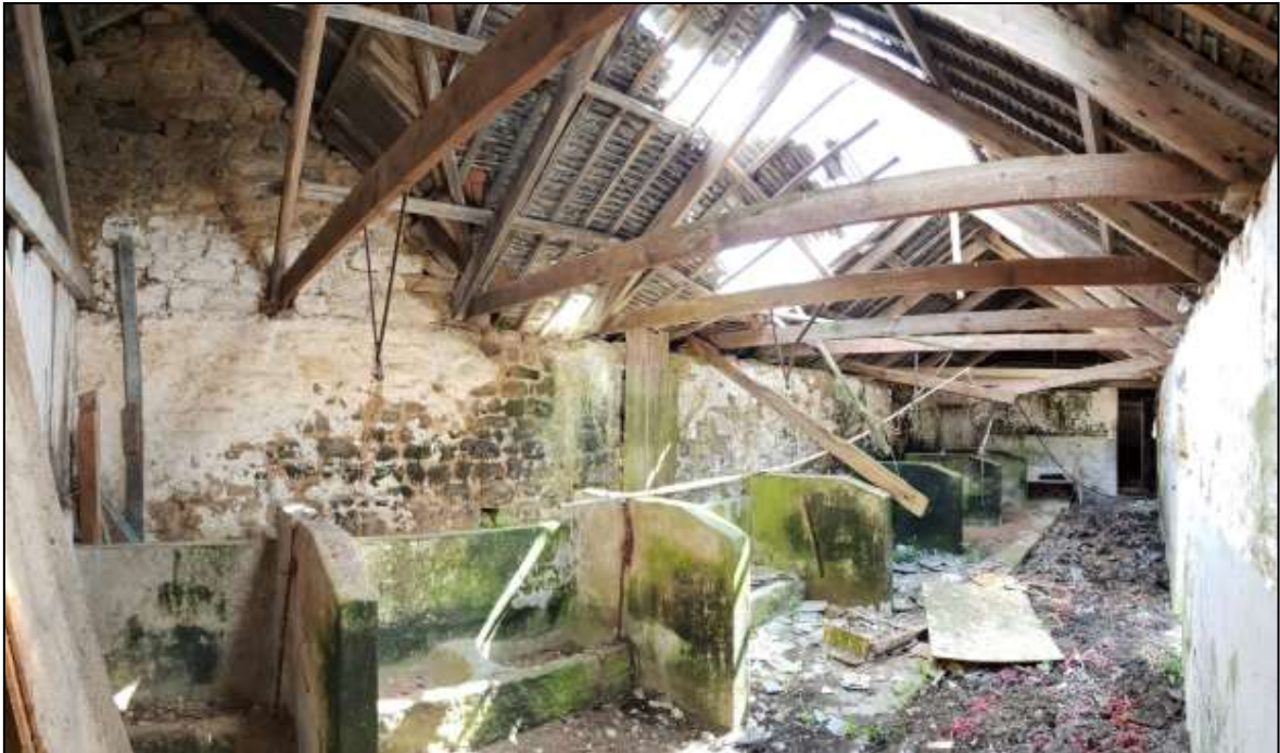
FIGURE 16: B4, PARTLY COLLAPSED 19 TH CENTURY ROOF AND MID-20 TH CENTURY CONCRETE CATTLE STALLS. NOTE ADDED INTERNAL GABLE OF B3 AT UPPER LEFT. VIEWED FROM THE NORTH.
