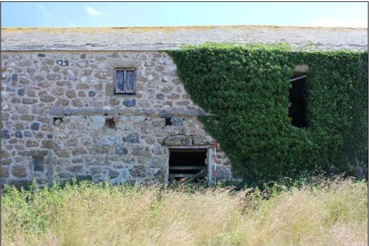
91. B9, THE CENTRAL SECTION OF THE NORTH-WEST ELEVATION; VIEWED FROM THE NORTH-WEST (SCALE 2M).
