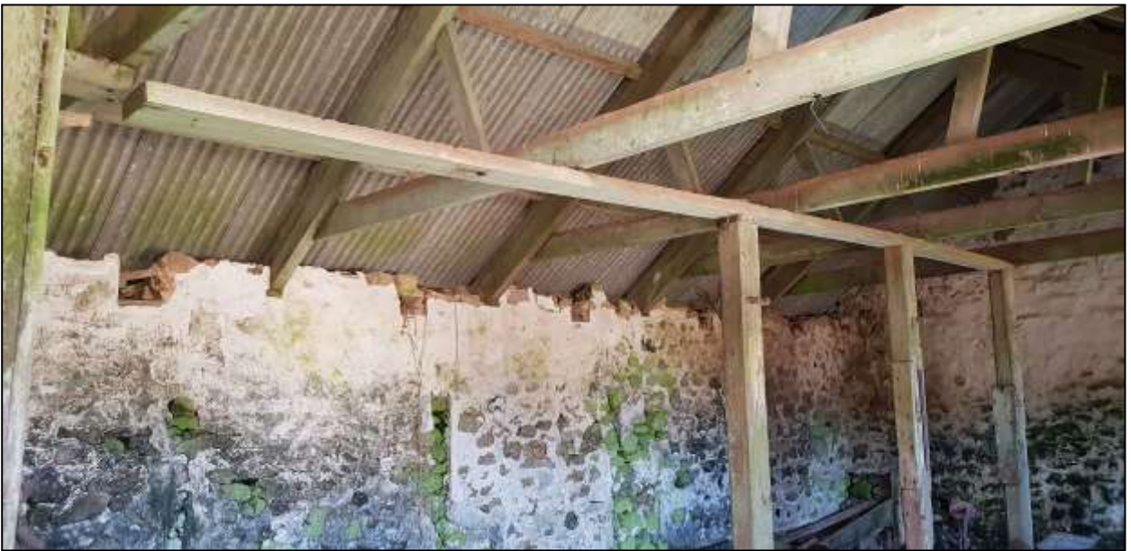
203. B10b INTERIOR, DETAIL OF THE OLD WOODEN STALLS AND ROOF STRUCTURE; VIEWED FROM THE SOUTH.
