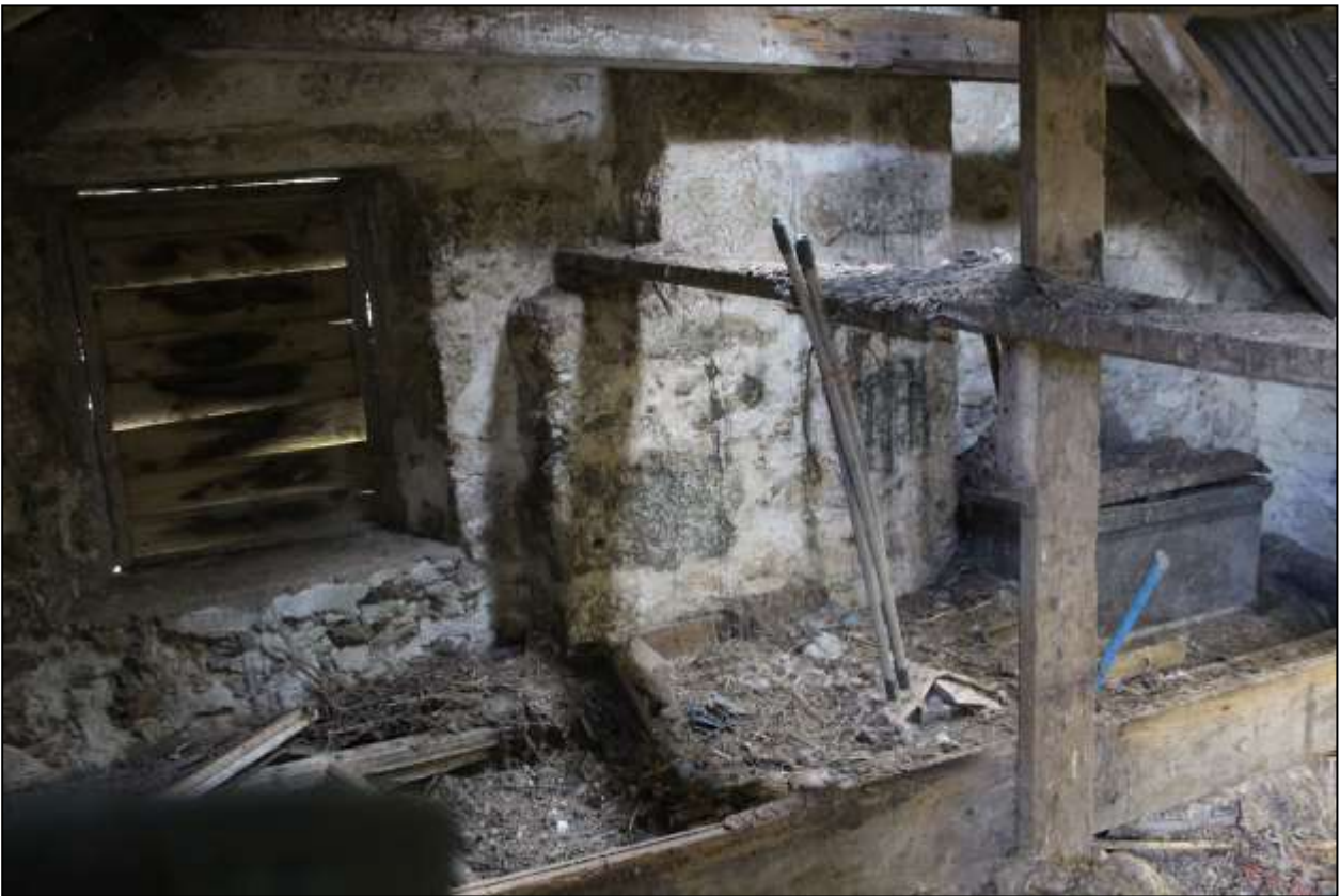
134. B3 FF INTERIOR, THE SOUTH-EAST WALL WITH FW2 AND STACK; VIEWED FROM THE NORTH-WEST.
