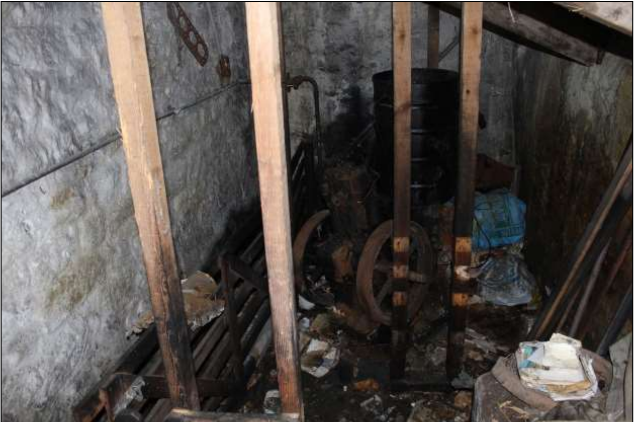
154. B6 INTERIOR, DETAIL OF THE 1HP ENGINE; VIEWED FROM THE SOUTH-EAST.
