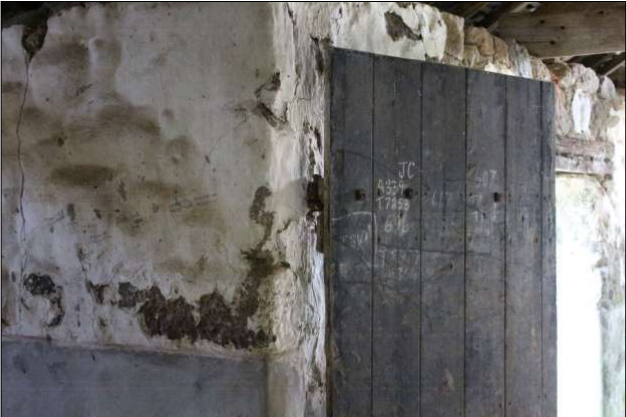
168. B7 INTERIOR, TALLY MARKS ON GD9 AND ADJACENT WALL; VIEWED FROM THE SOUTH.
