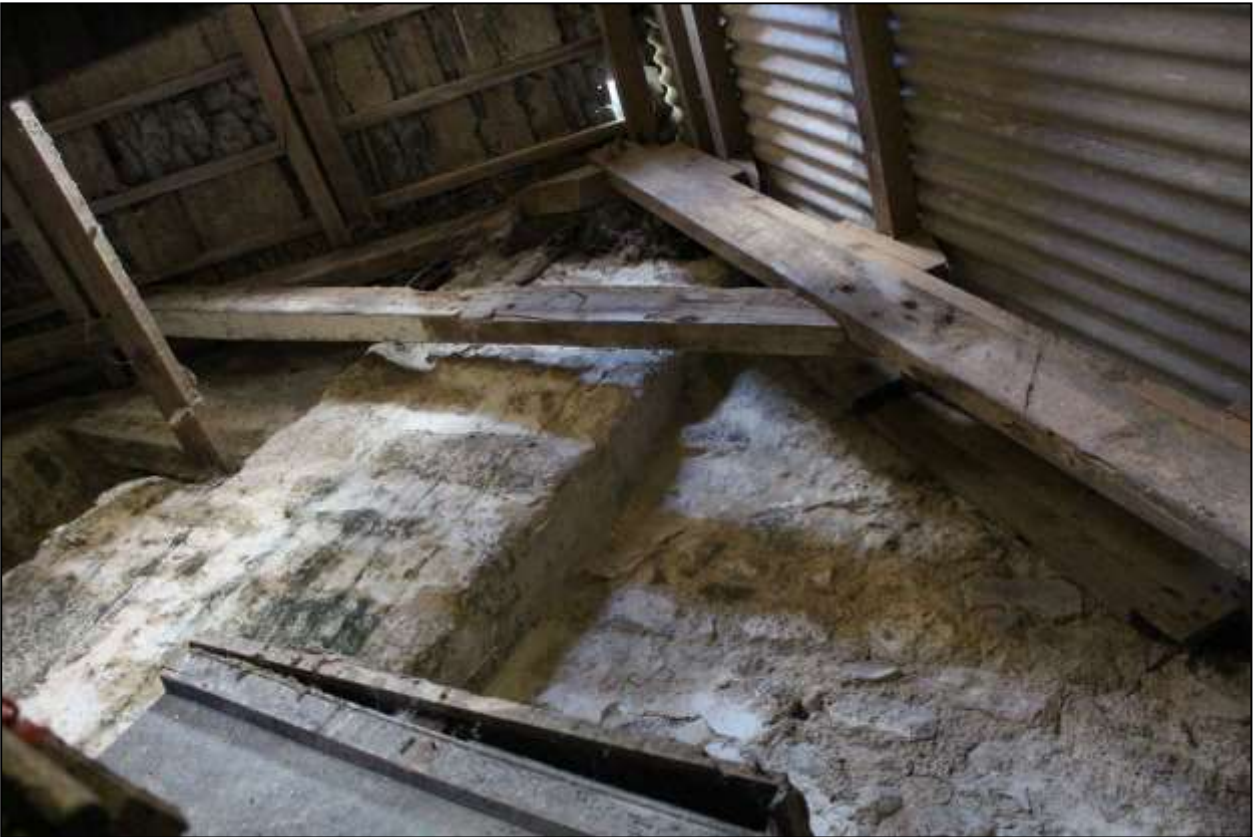
136. B3 FF INTERIOR, DETAIL OF THE SOUTH-EAST TRUSS; VIEWED FROM THE SOUTH.
