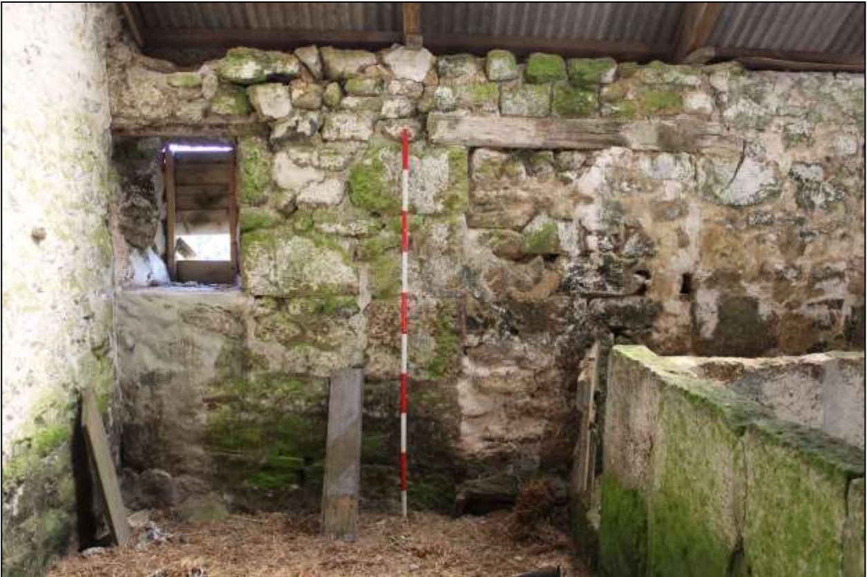
114. B1B INTERIOR, THE SOUTH-EAST WALL WITH GW2 AND BO2; VIEWED FROM THE NORTH-WEST (SCALE 2M).
