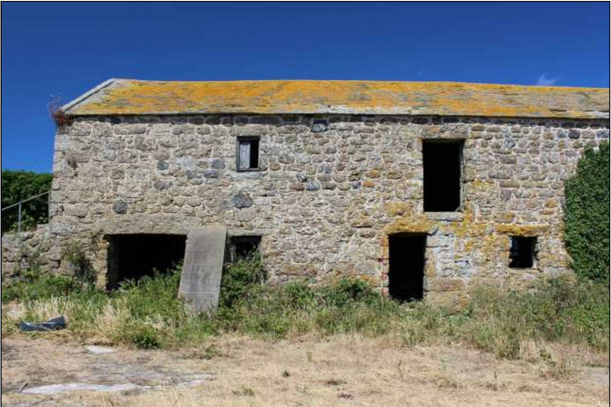
67. B9, THE SOUTH END OF THE SOUTH-EAST ELEVATION; VIEWED FROM THE SOUTH-EAST (SCALE 2M).
