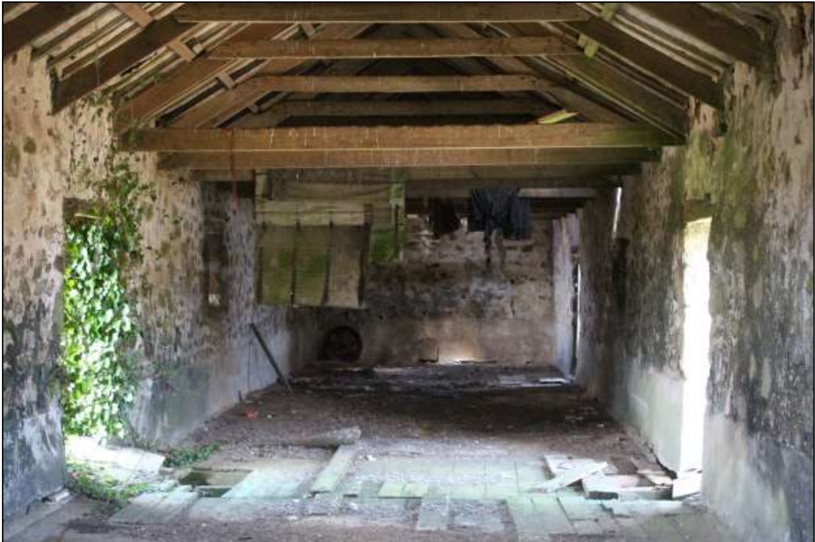
FIGURE 29: B9, FIRST-FLOOR THRESHING FLOOR BETWEEN THE OPPOSED THRESHING IN FOREGROUND AND MIXED A-FRAME AND TIEBEAM TRUSSES. NOTE CANVAS SHEETS FROM A REAPER/BINDER HUNG FROM TIEBEAMS TO REAR LEFT. VIEWED FROM THE SOUTH-WEST.
