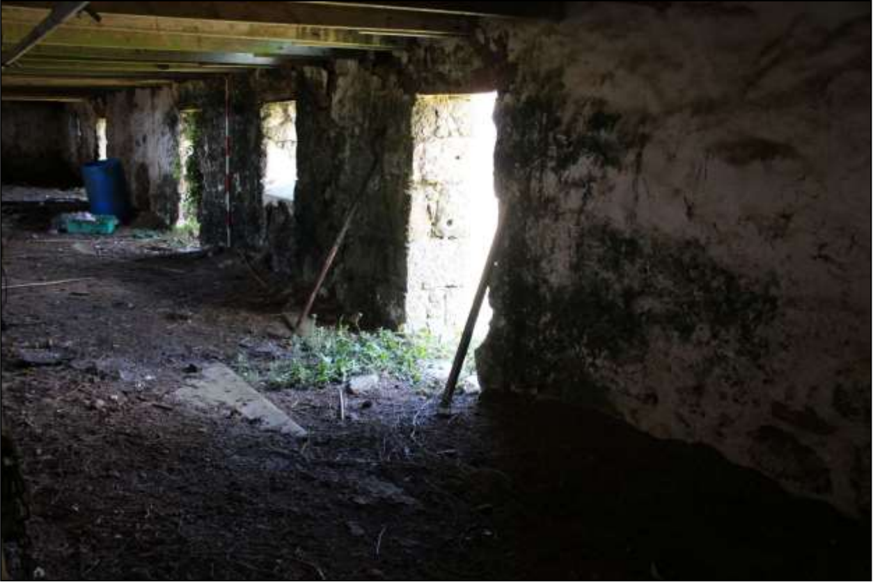
185. B9A GF INTERIOR, THE SOUTH-EAST WALL; VIEWED FROM THE WSW (SCALE 2M).
