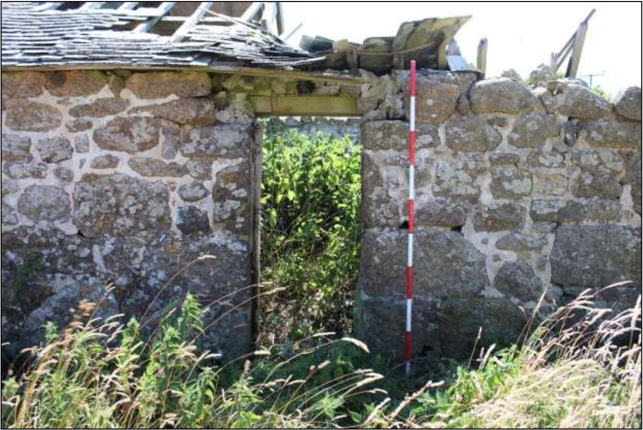
57. B1, NORTH-WEST ELEVATION, DETAIL OF GD22; VIEWED FROM THE NORTH-WEST (SCALE 2M).
