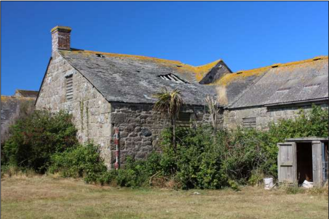
4. B3, NORTH-EAST AND SOUTH-EAST GABLE ELEVATION; VIEWED FROM THE EAST (SCALE 2M).
