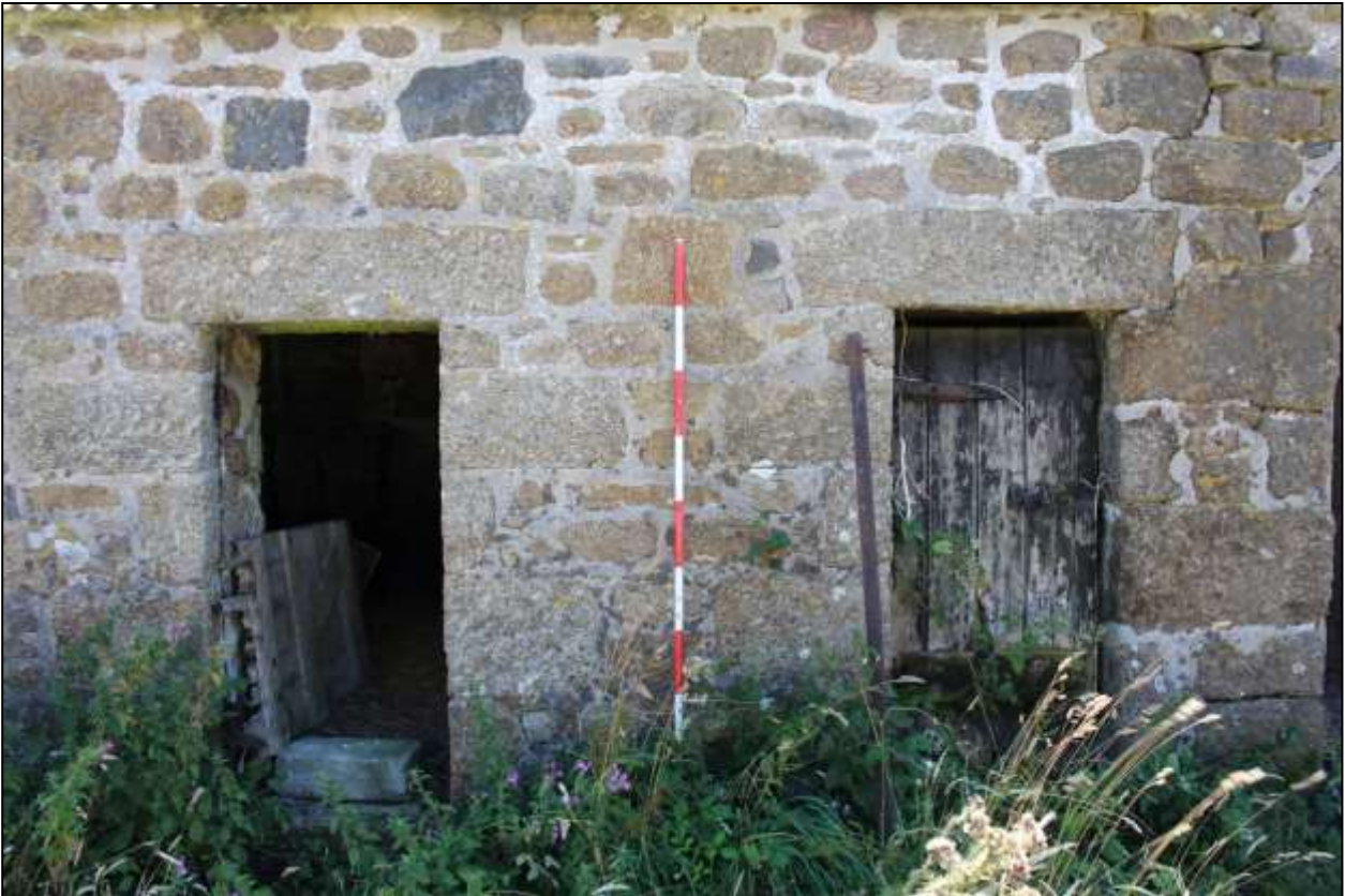
49. B2, NORTH-WEST ELEVATION, DETAIL OF GD15 AND GD16; VIEWED FROM THE NORTH-WEST (SCALE 2M).
