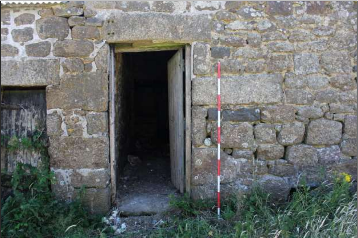
41. B4, NORTH-WEST ELEVATION, DETAIL OF GD12; VIEWED FROM THE NORTH-WEST (SCALE 2M).
