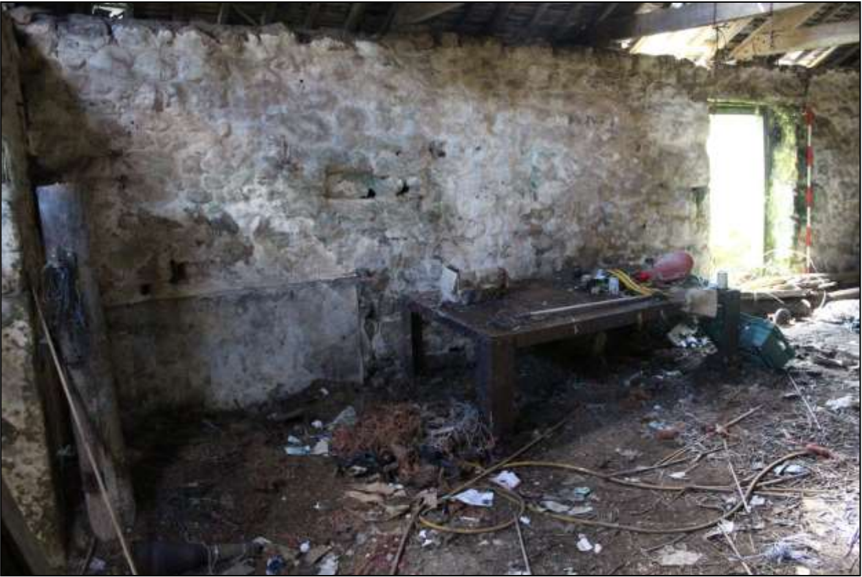
162. B7 INTERIOR, THE EAST END OF THE SOUTH-WEST WALL; VIEWED FROM THE NORTH-EAST (SCALE 2M).
