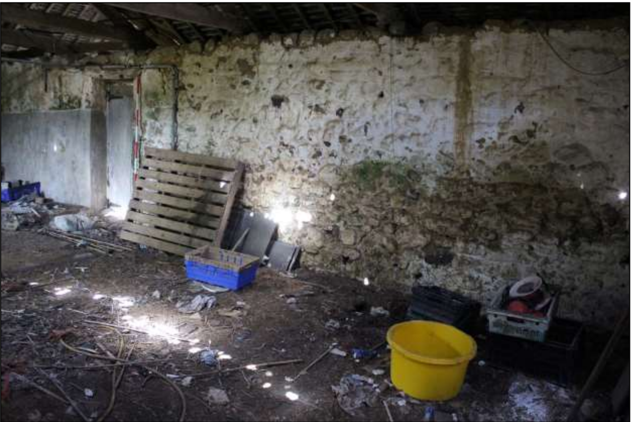
163. B7 INTERIOR, THE EAST END OF THE NORTH-EAST WALL; VIEWED FROM THE SOUTH (SCALE 2M).
