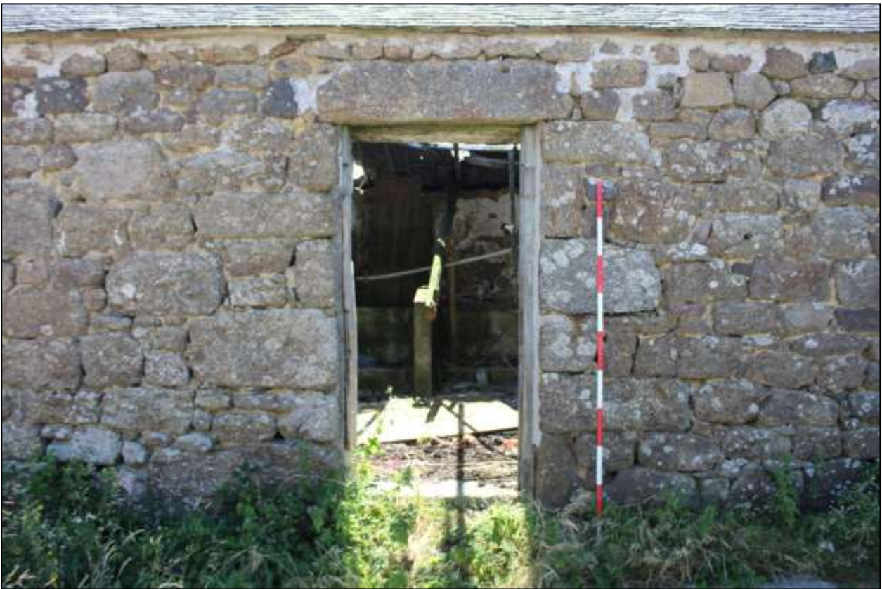
40. B4, NORTH-WEST ELEVATION, DETAIL OF GD11; VIEWED FROM THE NORTH-WEST (SCALE 2M).
