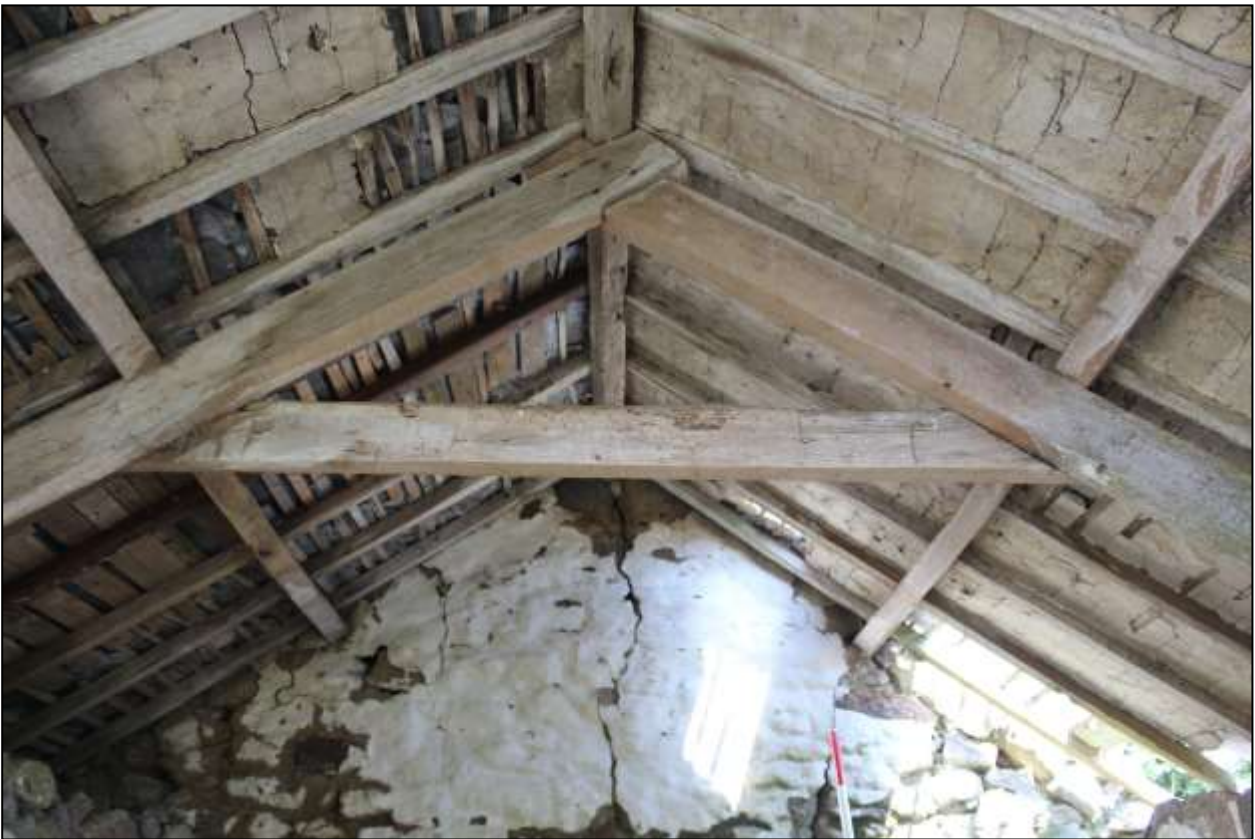
101. B1 INTERIOR, THE SURVIVING ROOF STRUCTURE OVER THE NORTHERN PART OF THE BUILDING; VIEWED FROM THE SOUTH-WEST.
