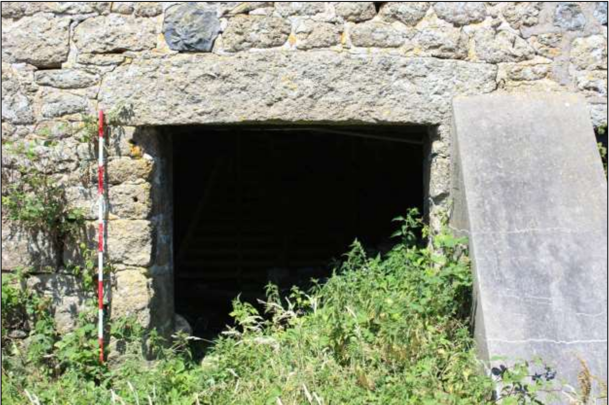
69. B9, SOUTH-EAST ELEVATION, DETAIL OF GD24; VIEWED FROM THE SOUTH-EAST (SCALE 2M).
