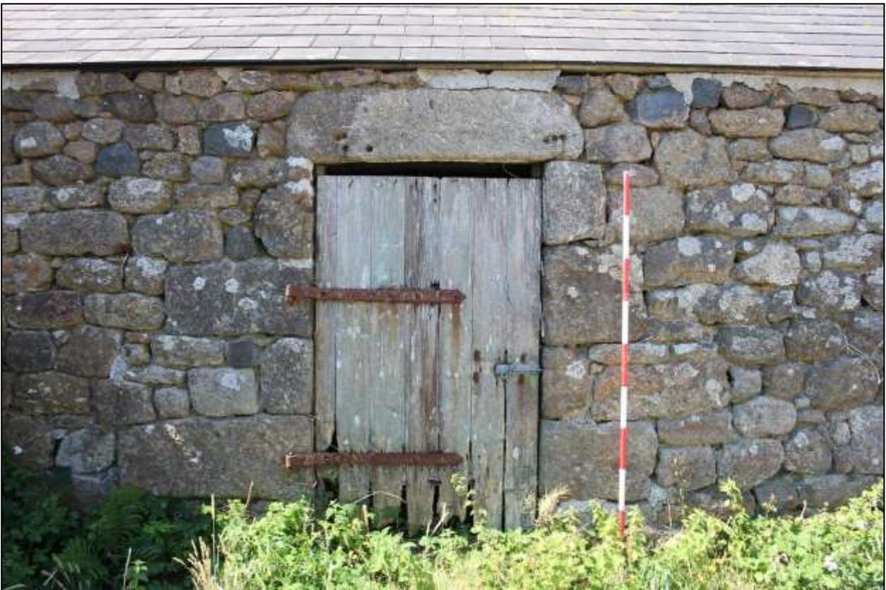
36. B7, NORTH-EAST ELEVATION, DETAIL OF GD7; VIEWED FROM THE NORTH-EAST (SCALE 2M).
