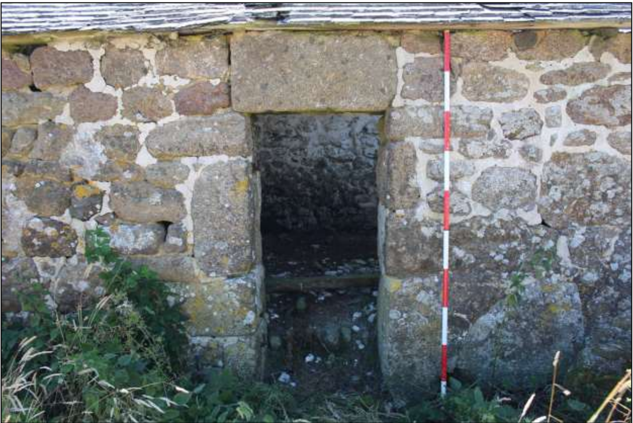
58. B1, NORTH-WEST ELEVATION, DETAIL OF GD23; VIEWED FROM THE NORTH-WEST (SCALE 2M).
