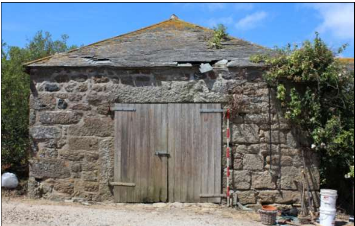
FIGURE 22: B7, THE SOUTH-EAST END, NOTE LARGE RE-USED GRANITE BLOCKS AND ENORMOUS GRANITE LINTEL; VIEWED FROM THE SOUTH-EAST (SCALE 2M).
