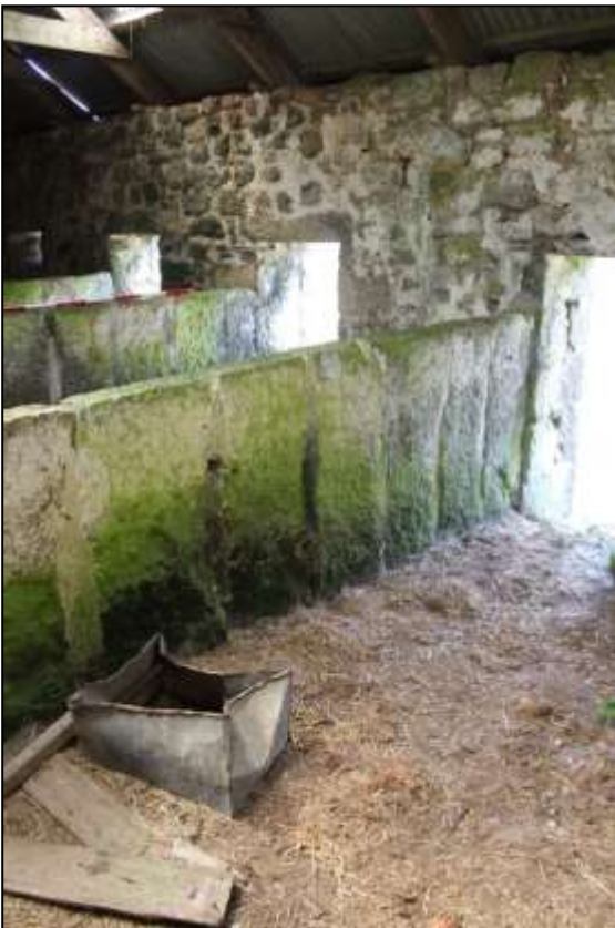
111. B1B INTERIOR, THE GRANITE SLAB PIGSTY WALLS; VIEWED FROM THE NORTH-EAST (SCALE 2M).
