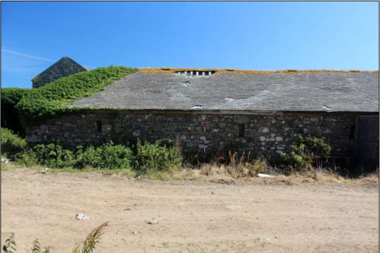
26. B7, THE WEST END OF THE SOUTH-WEST ELEVATION; VIEWED FROM THE SOUTH-WEST (SCALE 2M).
