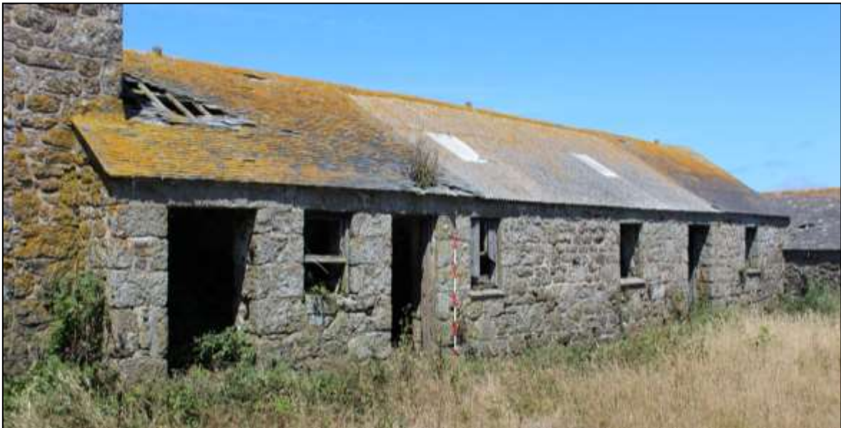
FIGURE 30: B10A (LEFT) AND B10B (RIGHT), SOUTH-EAST ELEVATION; VIEWED FROM THE SOUTH (SCALE 2M).
