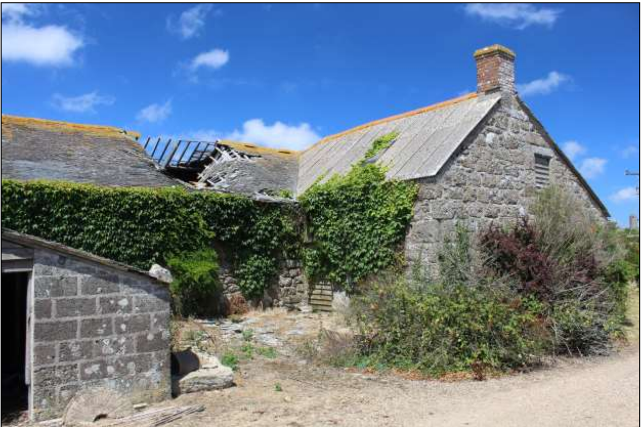
19. B3 AND B4, SOUTH-EAST AND SOUTH-WEST ELEVATIONS; VIEWED FROM THE SOUTH (SCALE 2M).
