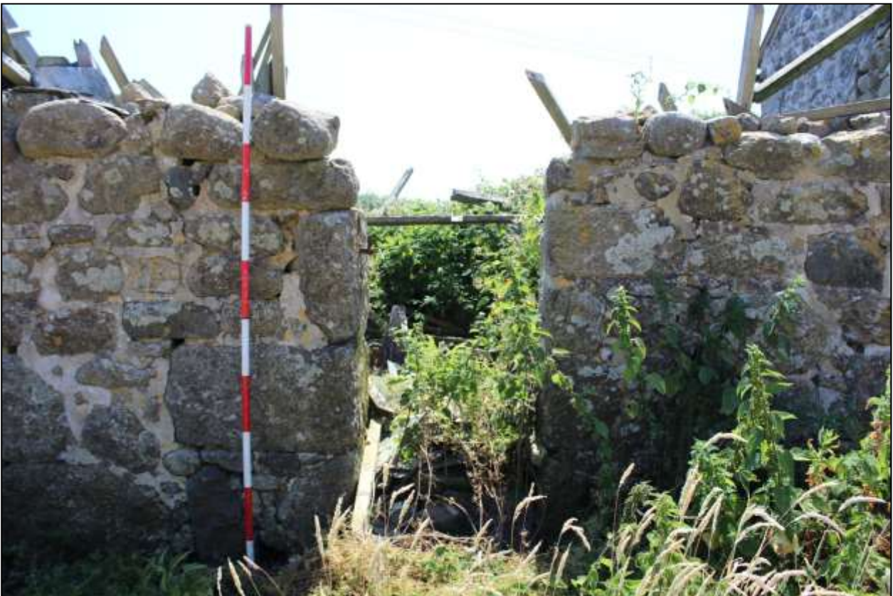
56. B1, NORTH-WEST ELEVATION, DETAIL OF GD21; VIEWED FROM THE NORTH-WEST (SCALE 2M).
