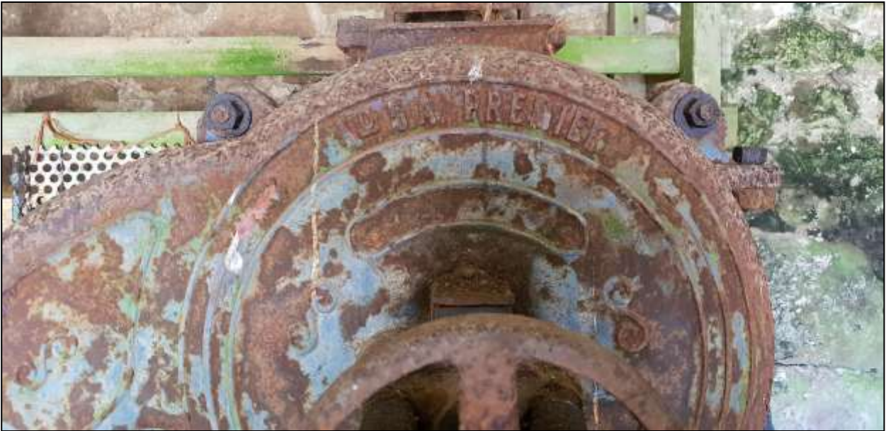
178. B9B GF INTERIOR, DETAIL OF BELT-DRIVEN ROLLER MILL; VIEWED FROM THE SOUTH-EAST.
