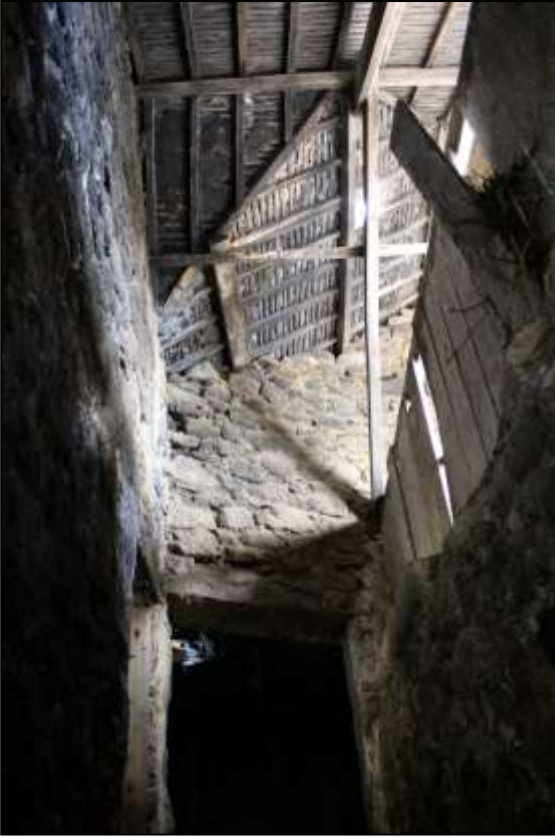
141. B4 INTERIOR, VIEW ABOVE THE CORRIDOR TO THE (SCORCHED?) UNDERSIDE OF THE ROOF; VIEWED FROM THE NORTH-WEST.
