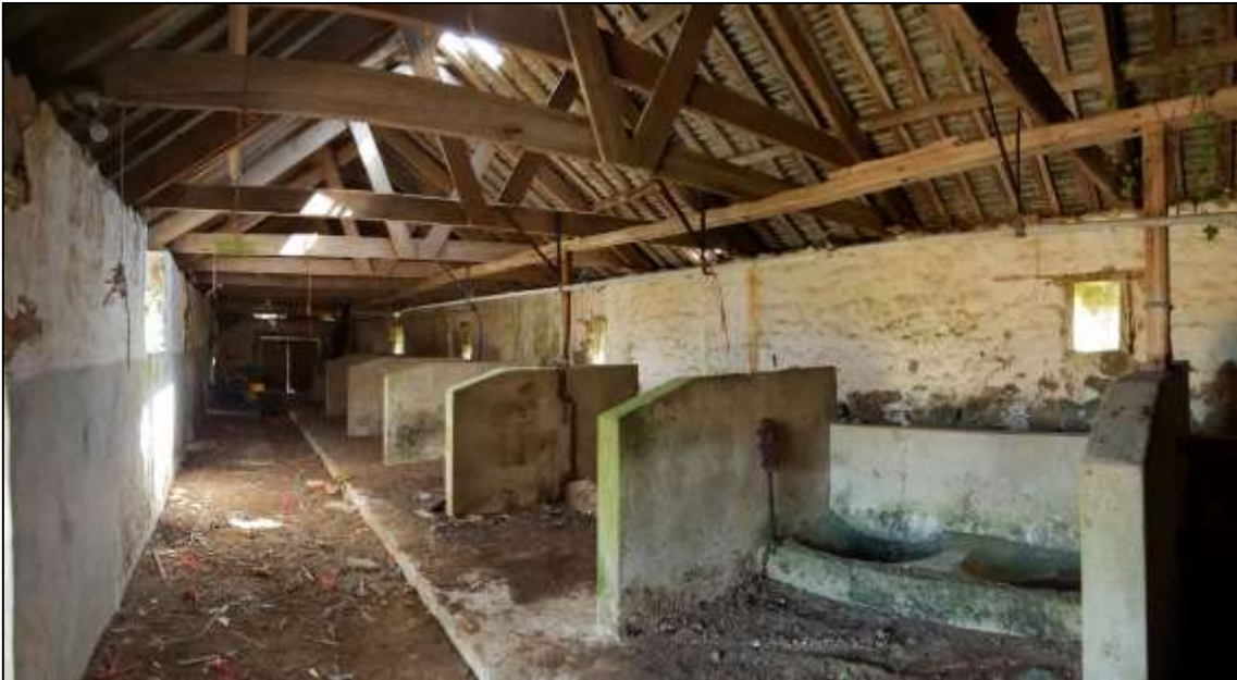
FIGURE 23: B7, 19 TH CENTURY TIEBEAM AND QUEEN-STRUT ROOF TRUSSES AND MID-20 TH CENTURY CATTLE STALLS; NOTE SUSPENDED GALVANISED STEEL PIPE SERVING DRINKERS. VIEWED FROM THE WEST.
