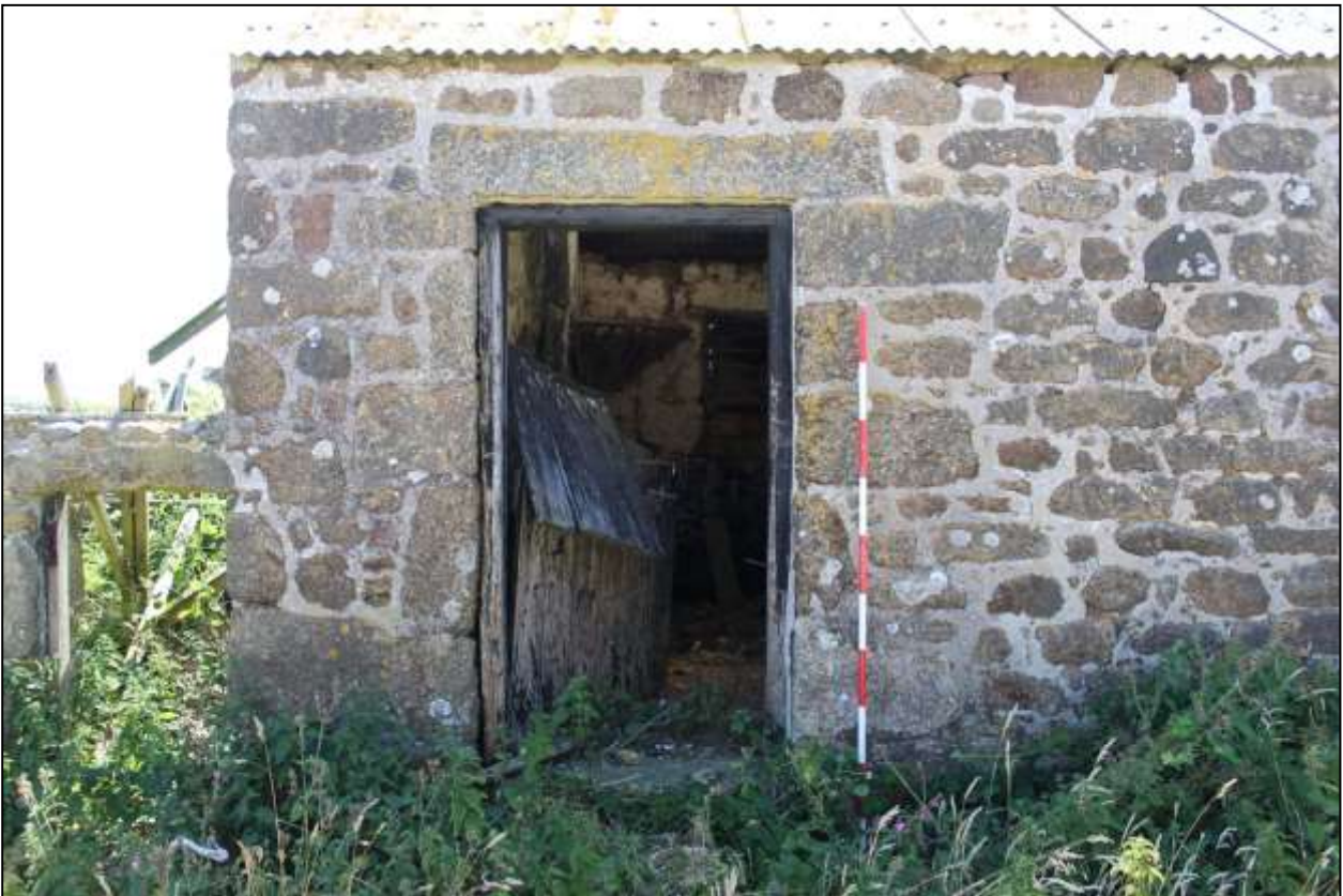
52. B2, NORTH-WEST ELEVATION, DETAIL OF GD19; VIEWED FROM THE NORTH-WEST (SCALE 2M).
