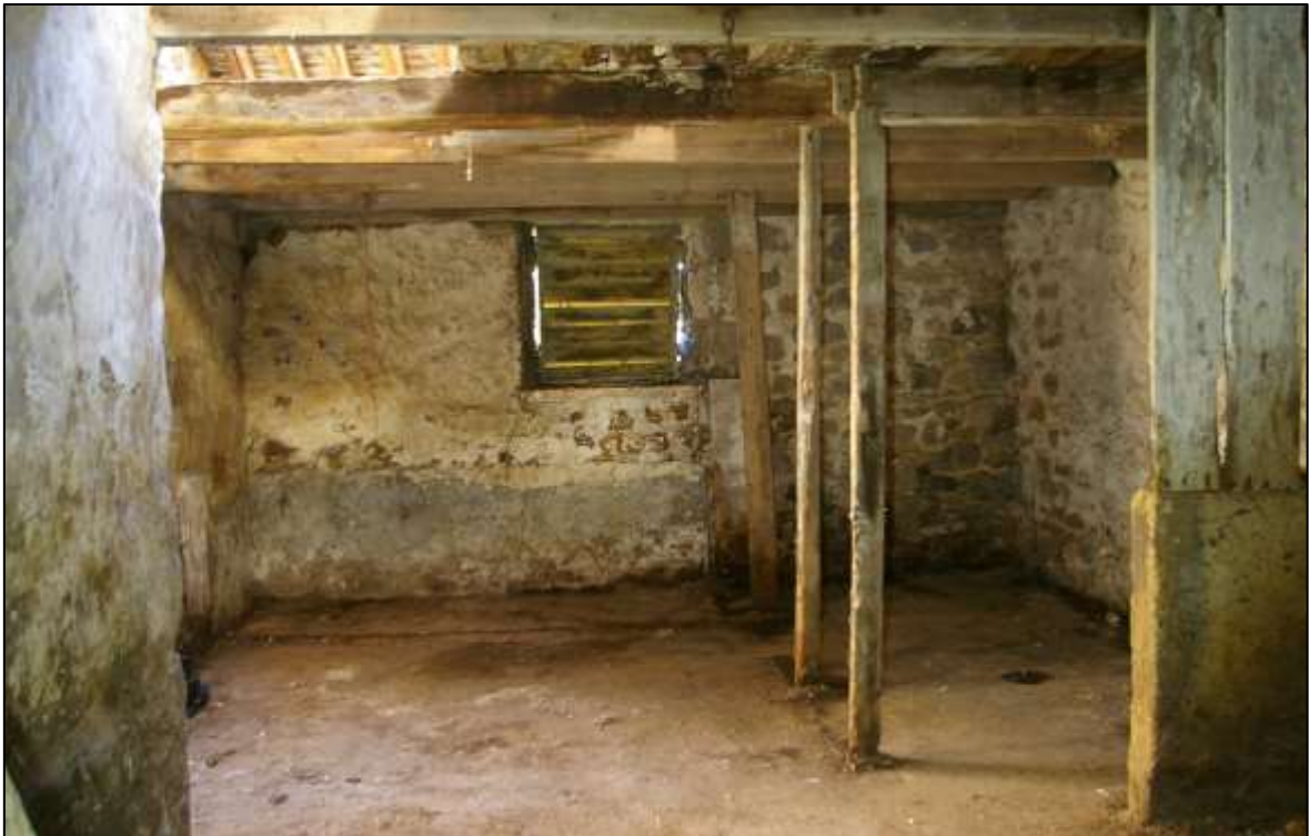
FIGURE 14: THE GROUND-FLOOR INTERIOR OF B3, CLEARED OF RUBBISH; THE FIREPLACE IS TO THE RIGHT OF THIS VIEW. VIEWED FROM THE SOUTH-WEST.
