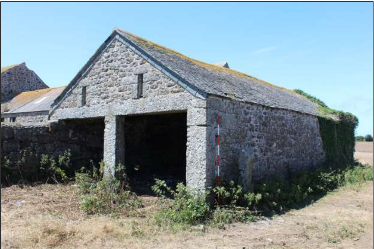
85. B11, SOUTH-EAST GABLE AND NORTH-EAST ELEVATIONS; VIEWED FROM THE EAST (SCALE 2M).
