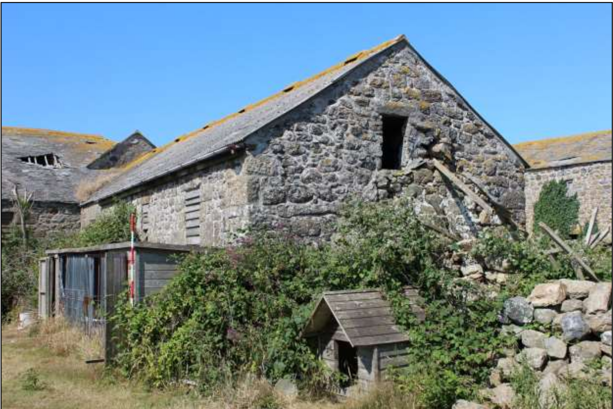
2. B2, SOUTH-EAST AND NORTH-EAST GABLE ELEVATION; VIEWED FROM THE EAST (SCALE 2M).
