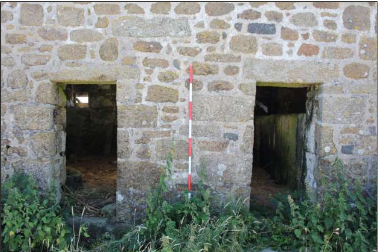
50. B2, NORTH-WEST ELEVATION, DETAIL OF GD17 AND GD18; VIEWED FROM THE NORTH-WEST (SCALE 2M).
