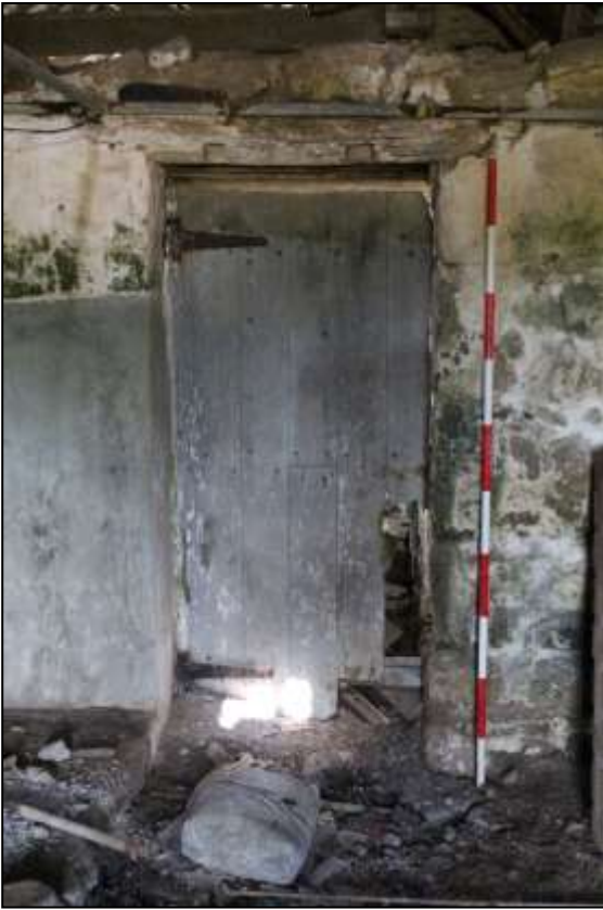
164. B7 INTERIOR, THE NORTH-EAST WALL WITH GD10; VIEWED FROM THE SOUTH-WEST (SCALE 2M).
