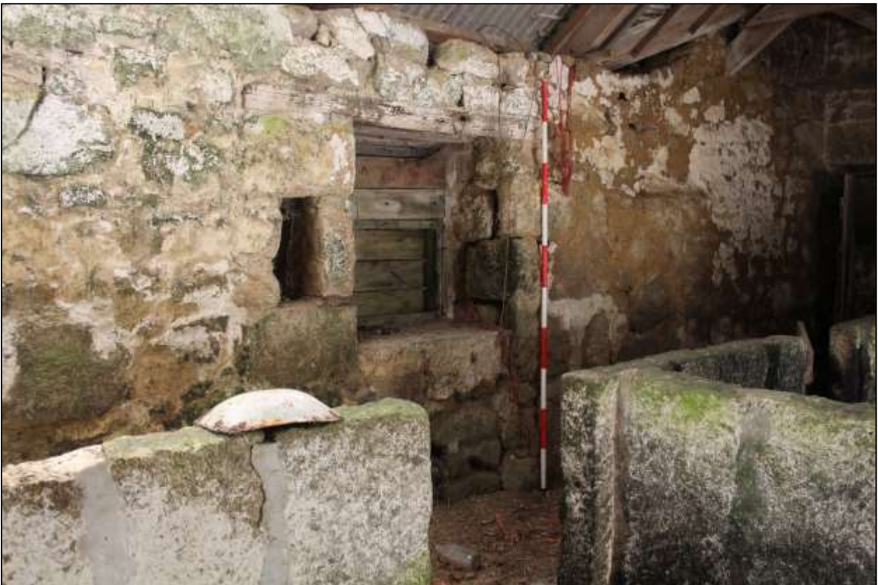
115. B1B INTERIOR, THE SOUTH-EAST WALL; BO3 WITH GW3 AND KEEPING PLACE; VIEWED FROM THE NORTH-WEST (SCALE 2M).
