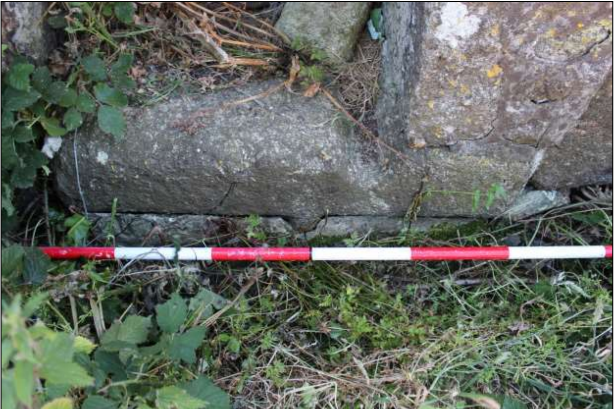
51. B2, NORTH-WEST ELEVATION, DETAIL OF GD18 SHOWING REUSED GRANITE WINDOW AS THRESHOLD; VIEWED FROM THE NORTH-WEST (SCALE 2M).
