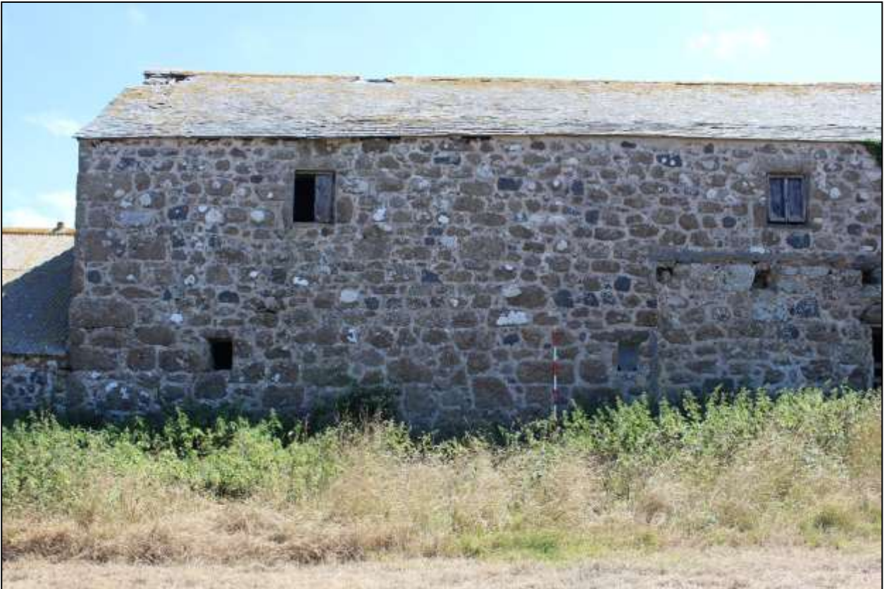
90. B9, THE NORTH END OF THE NORTH-WEST ELEVATION; VIEWED FROM THE NORTH-WEST (SCALE 2M).
