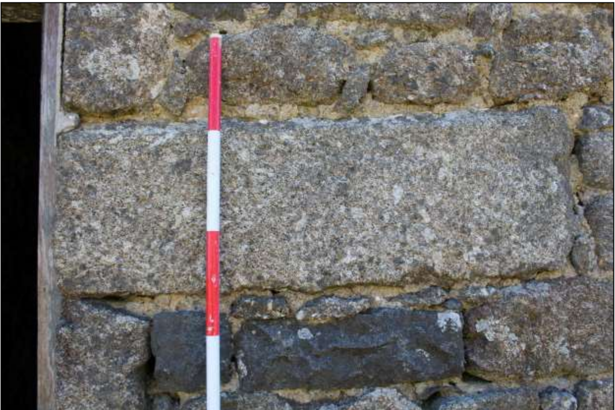
42. B4, NORTH-WEST ELEVATION, DETAIL OF REUSED GRANITE IN JAMB OF GD12; VIEWED FROM THE NORTH-WEST (SCALE 2M).
