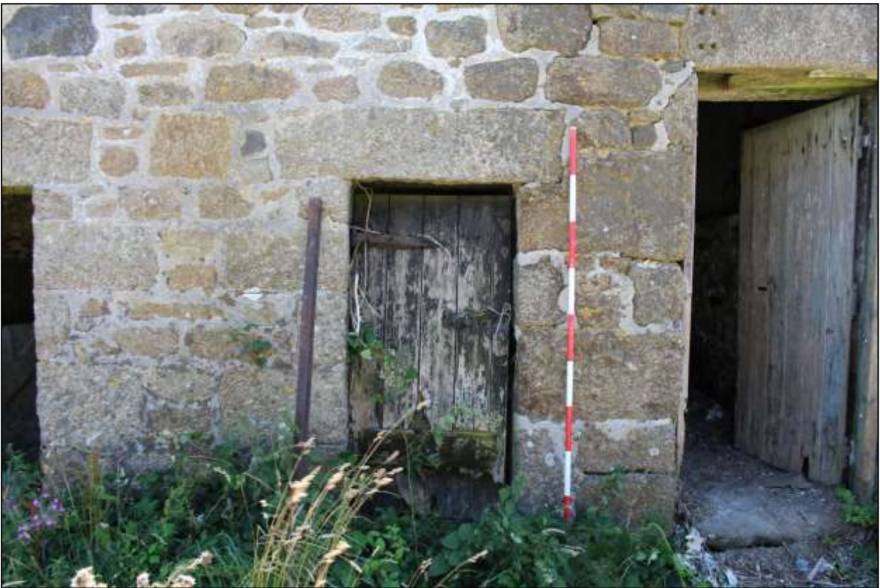
48. B2, NORTH-WEST ELEVATION, DETAIL OF GD15; VIEWED FROM THE NORTH-WEST (SCALE 2M).
