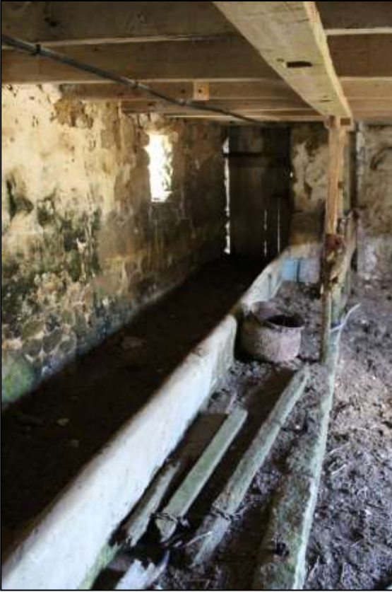
187. B9A GF INTERIOR, VIEW ALONG THE FEED PASSAGE TO GD32; VIEWED FROM THE SOUTH-WEST.
