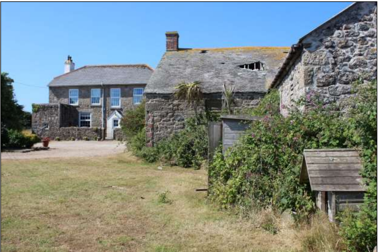
6. B3, NORTH-EAST ELEVATION WITH C19 FARMHOUSE IN BACKGROUND; VIEWED FROM THE NORTH-EAST (SCALE 2M).
