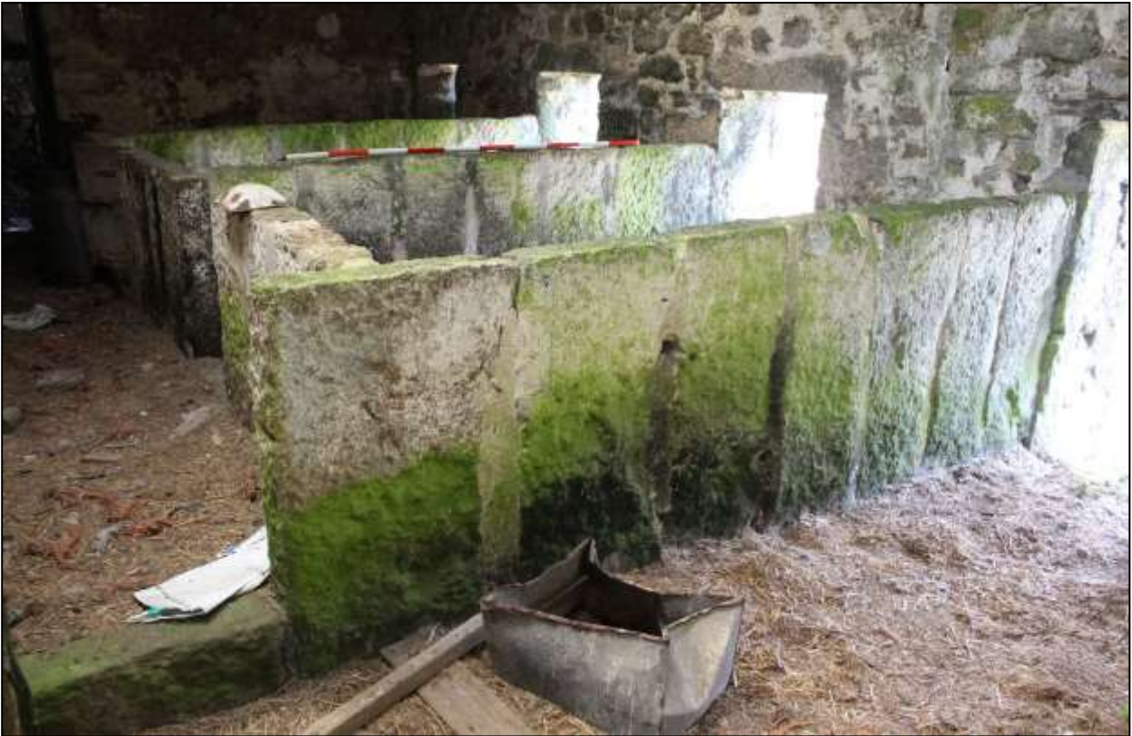
112. B1B INTERIOR, THE GRANITE SLAB PIGSTY WALLS; VIEWED FROM THE NORTH-EAST (SCALE 2M).
