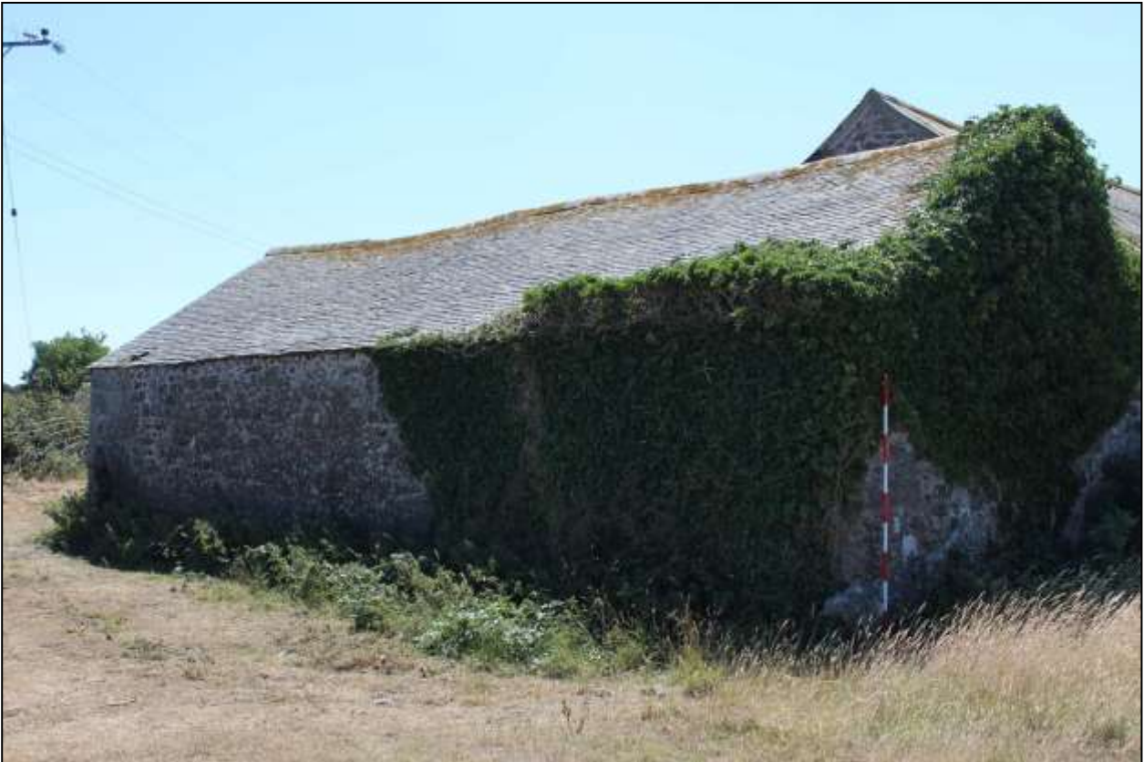
86. B11, NORTH-EAST AND NORTH-WEST GABLE ELEVATIONS; VIEWED FROM THE NORTH (SCALE 2M).
