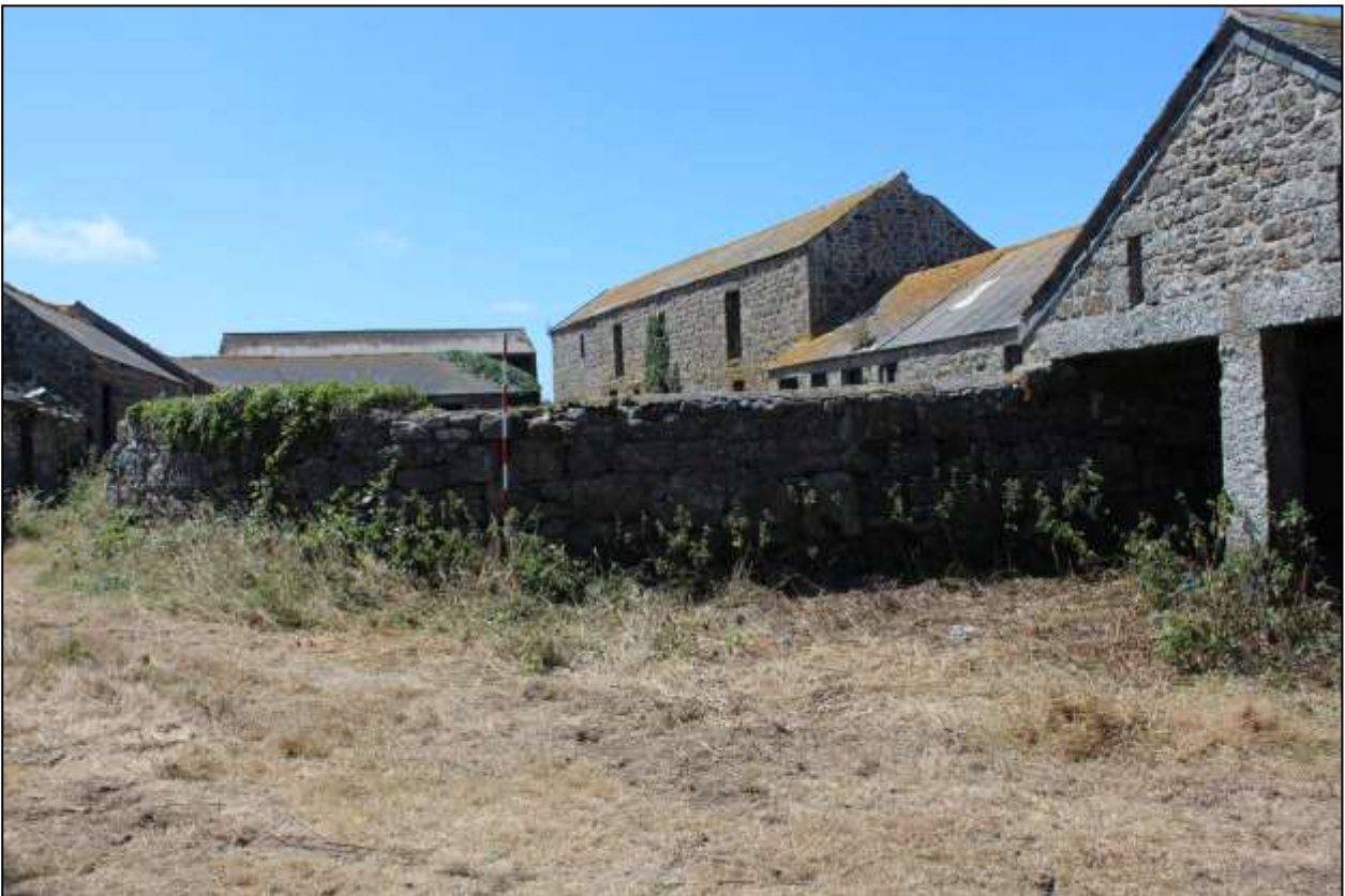
83. THE NORTH YARD WALL WITH B9 BEYOND; VIEWED FROM THE NORTH (SCALE 2M).
