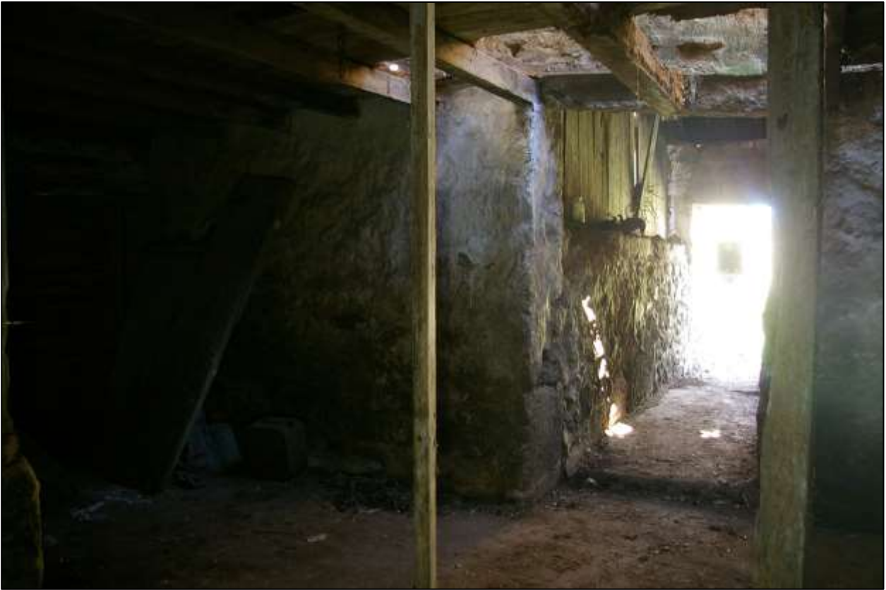
124. B3 GF INTERIOR, CLEARED OF RUBBISH, LOOKING BACK ALONG THE PASSAGE IN B4; VIEWED FROM THE SOUTH-EAST.
