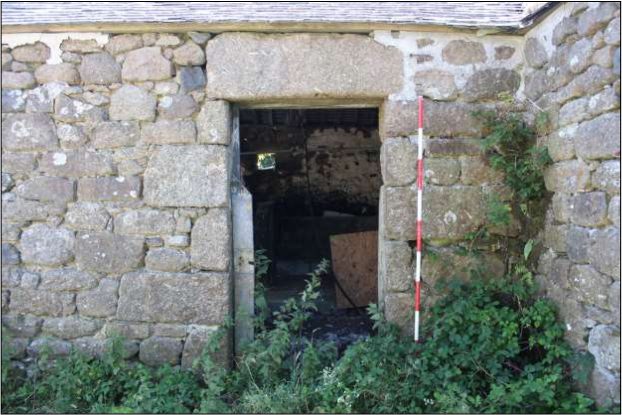
39. B4, NORTH-WEST ELEVATION, DETAIL OF GD8; VIEWED FROM THE NORTH-WEST (SCALE 2M).
