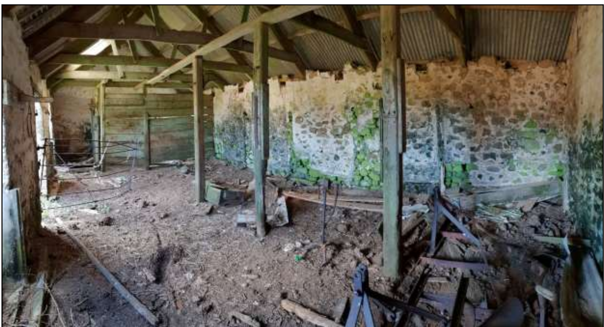
FIGURE 32: B10B, INTERIOR. NOTE THE POSTS SUPPORTING STALL DIVIDERS, SINCE LOST EXCEPT TO THE SOUTH-WEST END. WOODEN TACK RAIL ON WALL TO UPPER LEFT AND 19 TH CENTURY WROUGHT IRON GATE AT CENTRE LEFT. VIEWED FROM THE EAST.
