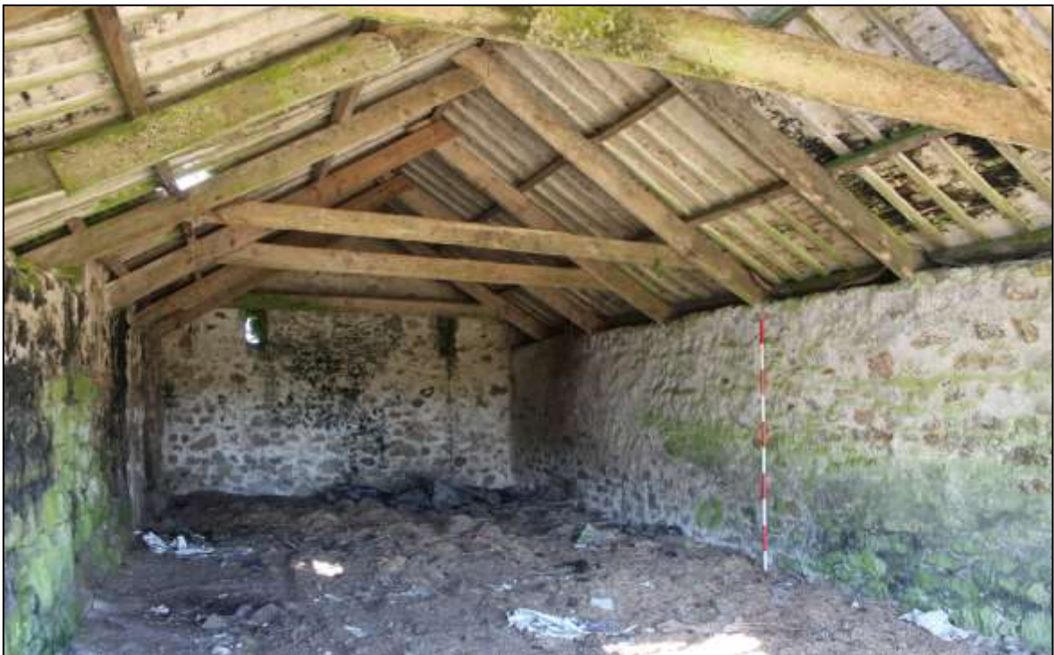
FIGURE 35: B11, INTERIOR, NOTE PLASTER TORCHING BETWEEN COMMON RAFTERS; VIEWED FROM THE SSE (SCALE 2M).
