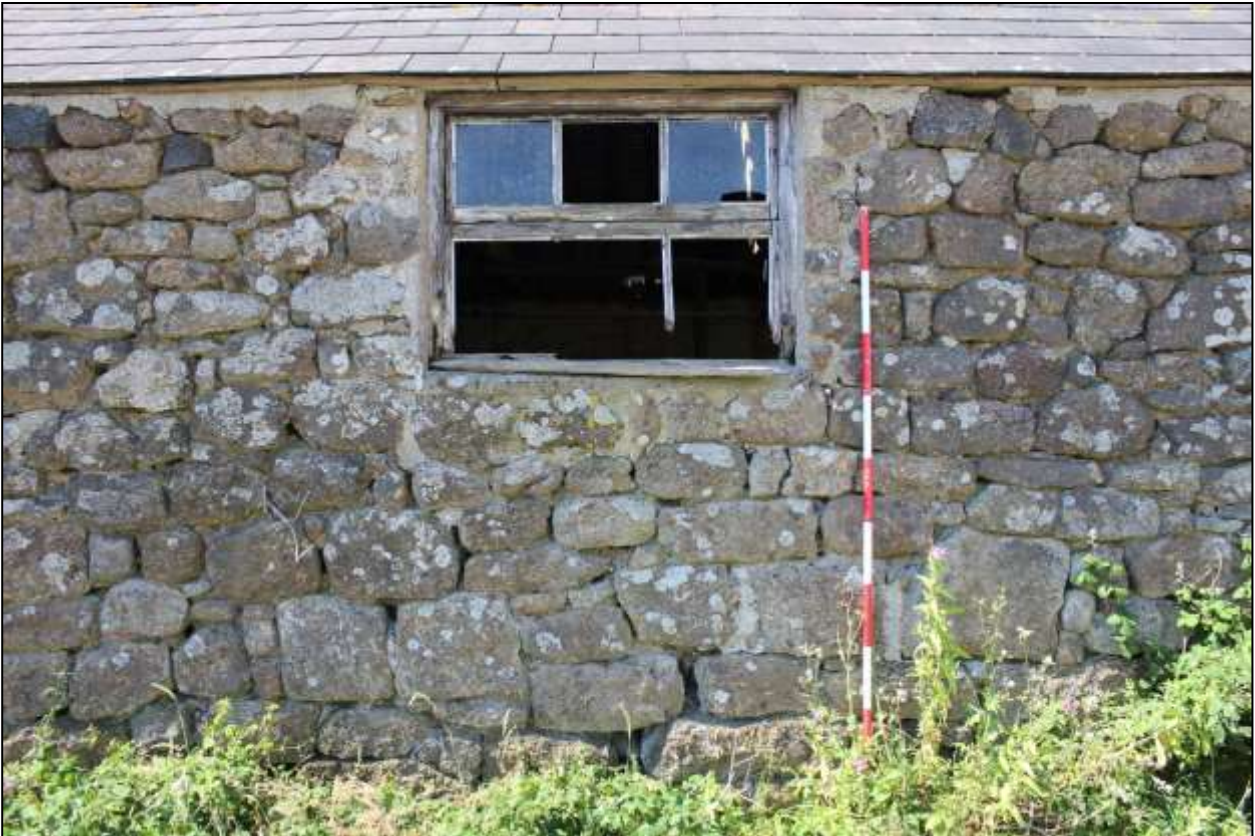
35. B7, NORTH-EAST ELEVATION, DETAIL OF GW11; VIEWED FROM THE NORTH-EAST (SCALE 2M).
