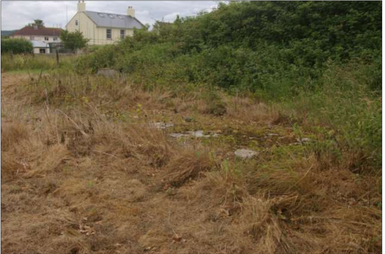
Field 2; the concrete structure at the southern end of Field 2; viewed from the west, looking east.
