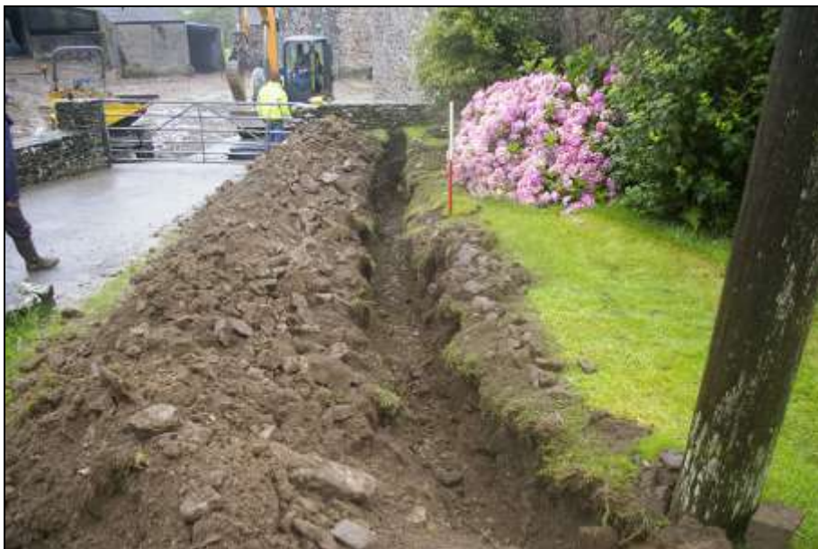
FIGURE 4: SOUTHERN 10M OF SERVICE TRENCH THROUGH GARDEN; VIEWED FROM THE SOUTH (1M SCALE).
