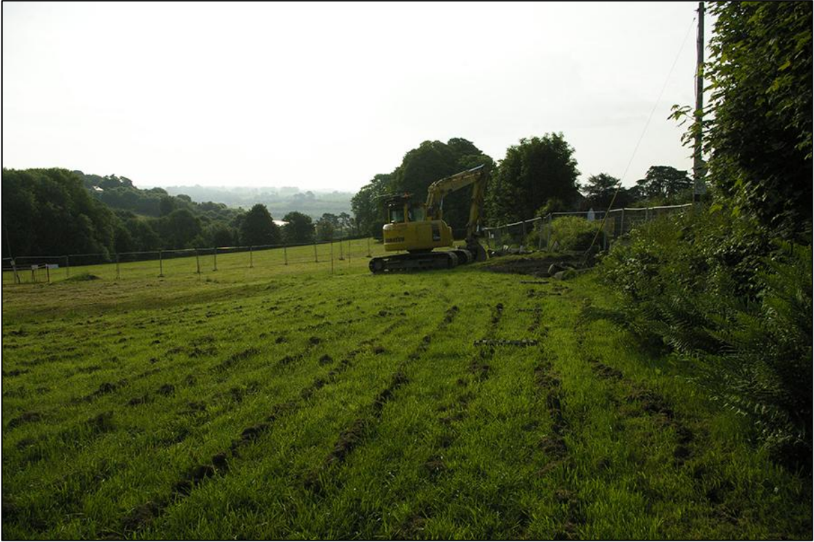
3. SITE VIEW PRE-EXCAVATION, SHOWING NATURAL SLOPE OF THE GROUND; VIEWED FROM THE WEST (NO SCALE).
