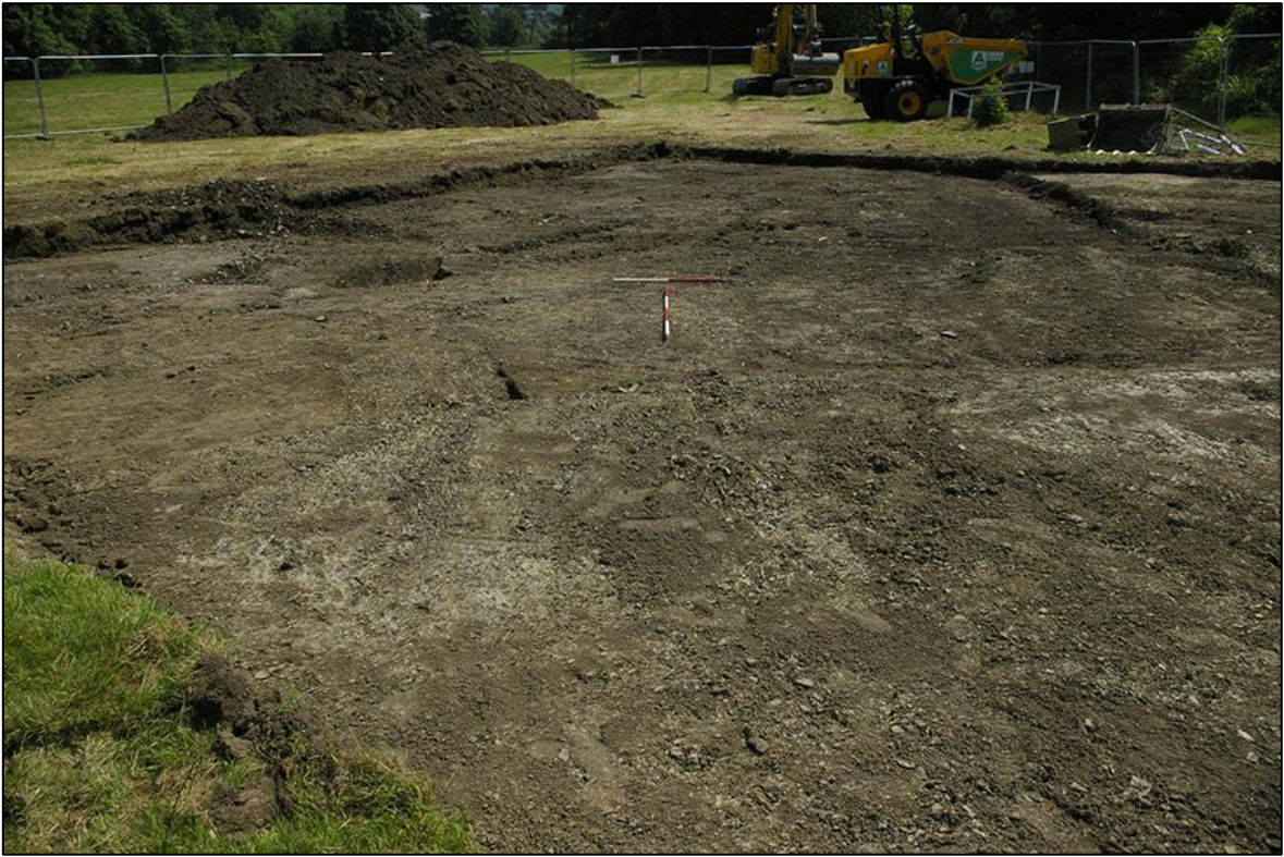
7. POST-EXCAVATION VIEW OF SITE, EAST END; VIEWED FROM THE NORTH-WEST (1M & 2M SCALES).
