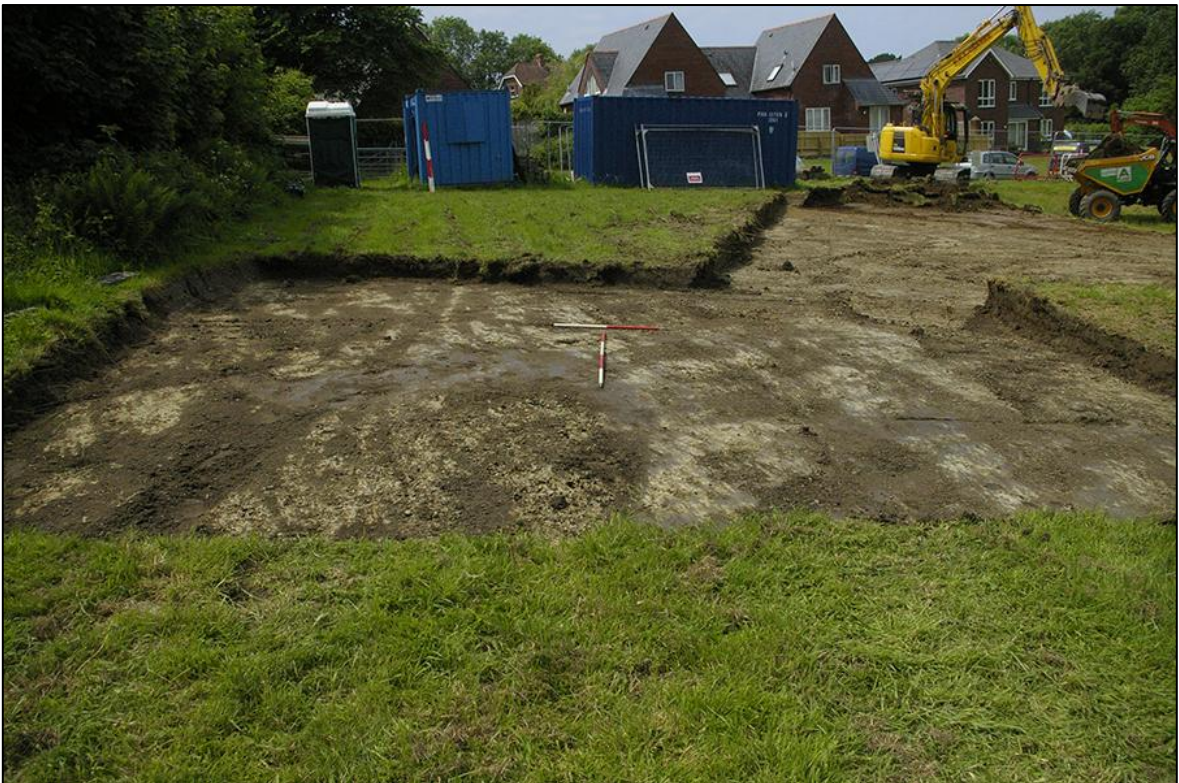
10. POST-EXCAVATION VIEW OF SITE, SOUTHERN EDGE; VIEWED FROM THE EAST (1M & 2M SCALES).
