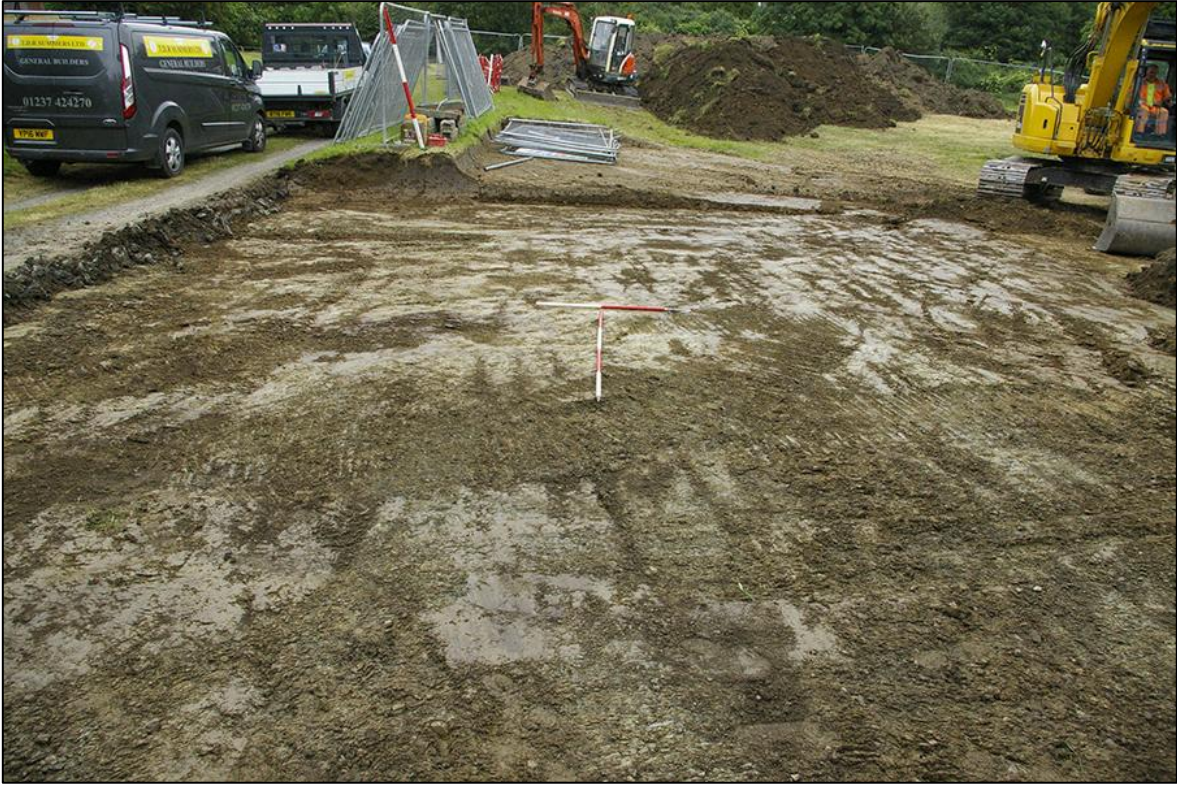
11. POST-EXCAVATION VIEW OF SITE, WEST END; VIEWED FROM THE SOUTH (1M & 2M SCALES).
