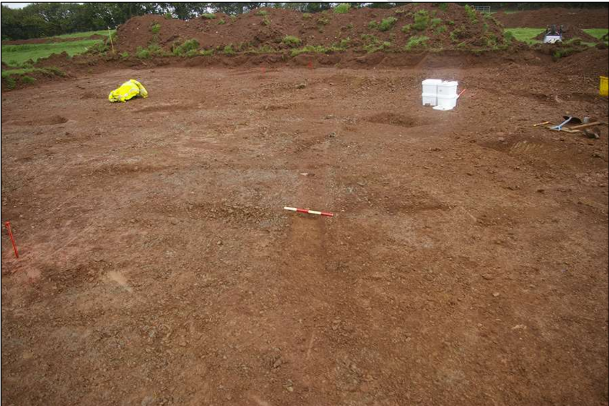
45. GULLY [814]A AND MID-EXCAVATION SITE SHOT; VIEWED FROM THE SOUTH-EAST (0.40M SCALE).
