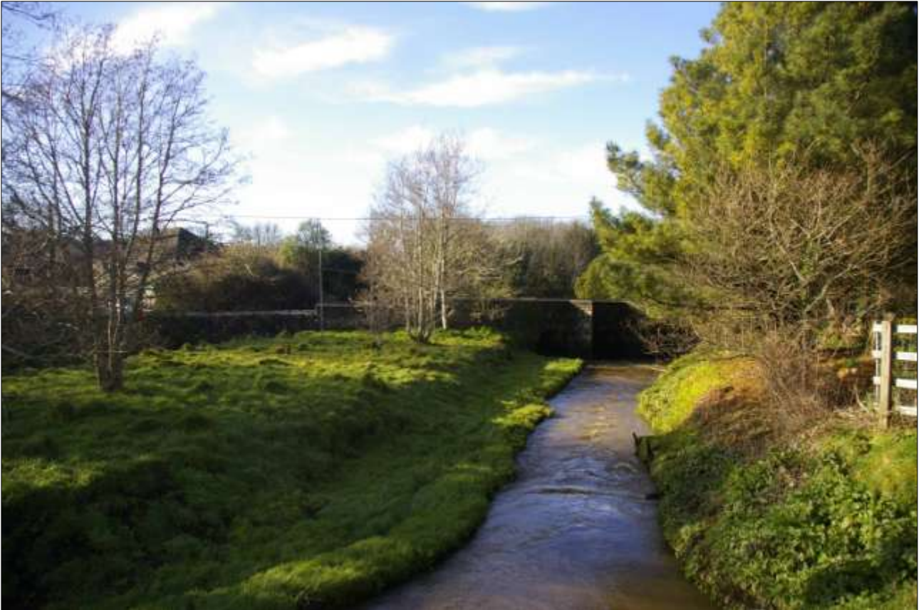
15. VIEW OF ST ERTH BRIDGE CROSSING THE RIVER; VIEWED FROM THE SOUTH.
