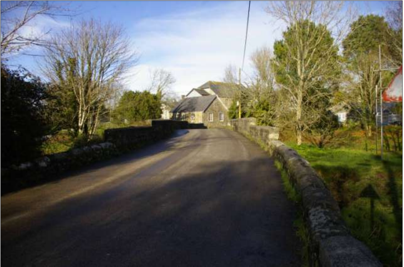
17. VIEW ALONG THE EASTERN SECTION OF ST ERTH BRIDGE; VIEWED FROM THE WEST.
