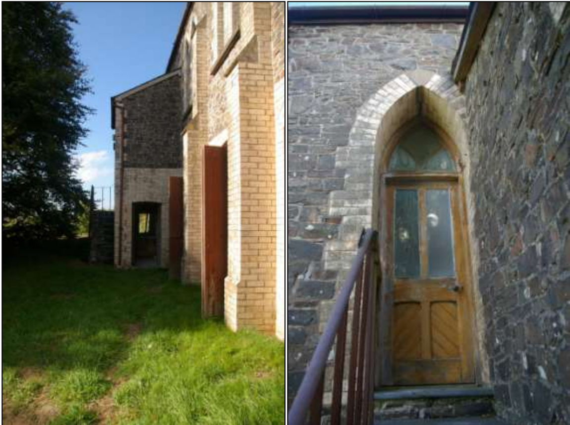
23. LEFT: THE EAST ELEVATION OF THE SMALL PROJECTING SERVICE BLOCK, WITH 2M SCALE; FROM THE EAST.
