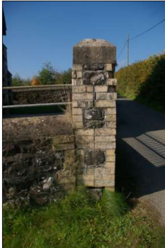
19. VIEW OF HOW THE EAST SIDE WALLS AND RAILINGS ABUT, THE SIDE WALLS SEEMING TO BE LATER, POSSIBLY A REPAIR; FROM THE EAST.
