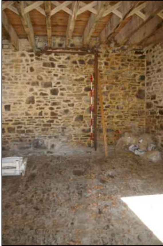
50. THE BOILER PIPES, WHERE THEY BREACH THE WALL OF THE CARRIAGE HOUSE, WITH 2M SCALE; FROM THE SOUTH.
