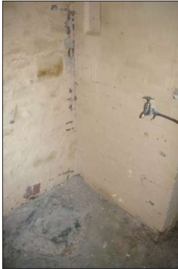
122. SCARRING ON THE FLOOR OF THE SERVICES BLOCK SHOWING REMOVED FITMENTS AND A TAP FOR RUNNING WATER; FROM THE SOUTH-EAST.
