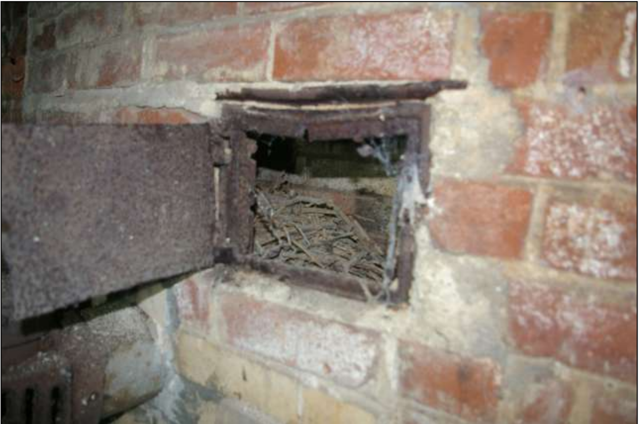
32. VIEW THROUGH THE HATCH SHOWING THE FLUE BLOCKED WITH JACKDAW NESTS; FROM THE NORTH-WEST.
