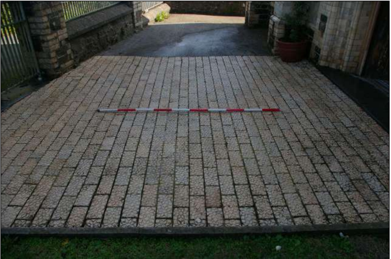
7. THE CAST CERAMIC BRICK RELIEF MOULDED PAVEMENT LEADING TO THE FRONT DOOR; FROM THE WEST.
