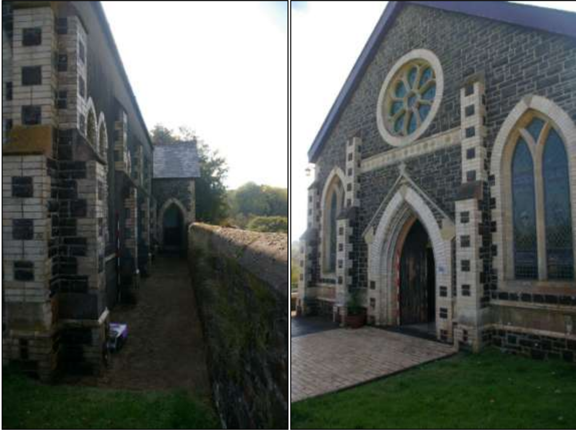
4. LEFT: THE WEST ELEVATION OF THE CHAPEL AND THE VESTRY BEYOND, WITH 2M SCALE; FROM THE NORTH.
