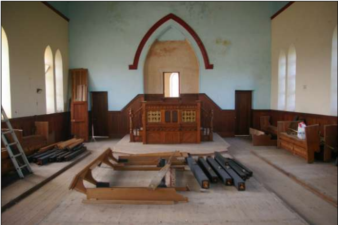
FIGURE 3: THE SOUTH WALL OF THE CHAPEL, WITH ALCOVE BEHIND THE PULPIT WITH FINE HOODMOULD OVER; FROM THE NORTH.
