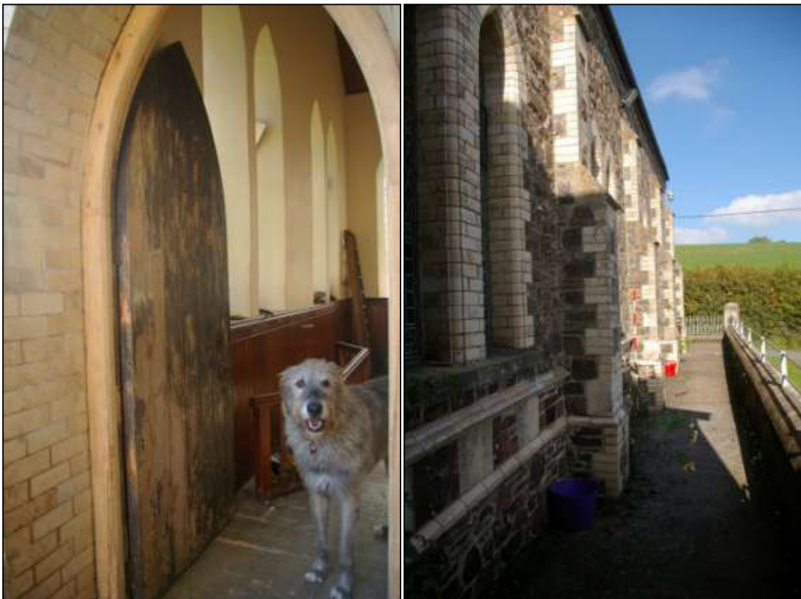
15. LEFT: THE EAST DOOR OPENED, SHOWING VIEW INTO THE COMMUNITY HALL; FROM THE NORTH. 16. RIGHT: VIEW BACK ALONG THE EAST ELEVATION, WITH 2M SCALE; FROM THE SOUTH, SOUTH-EAST.
