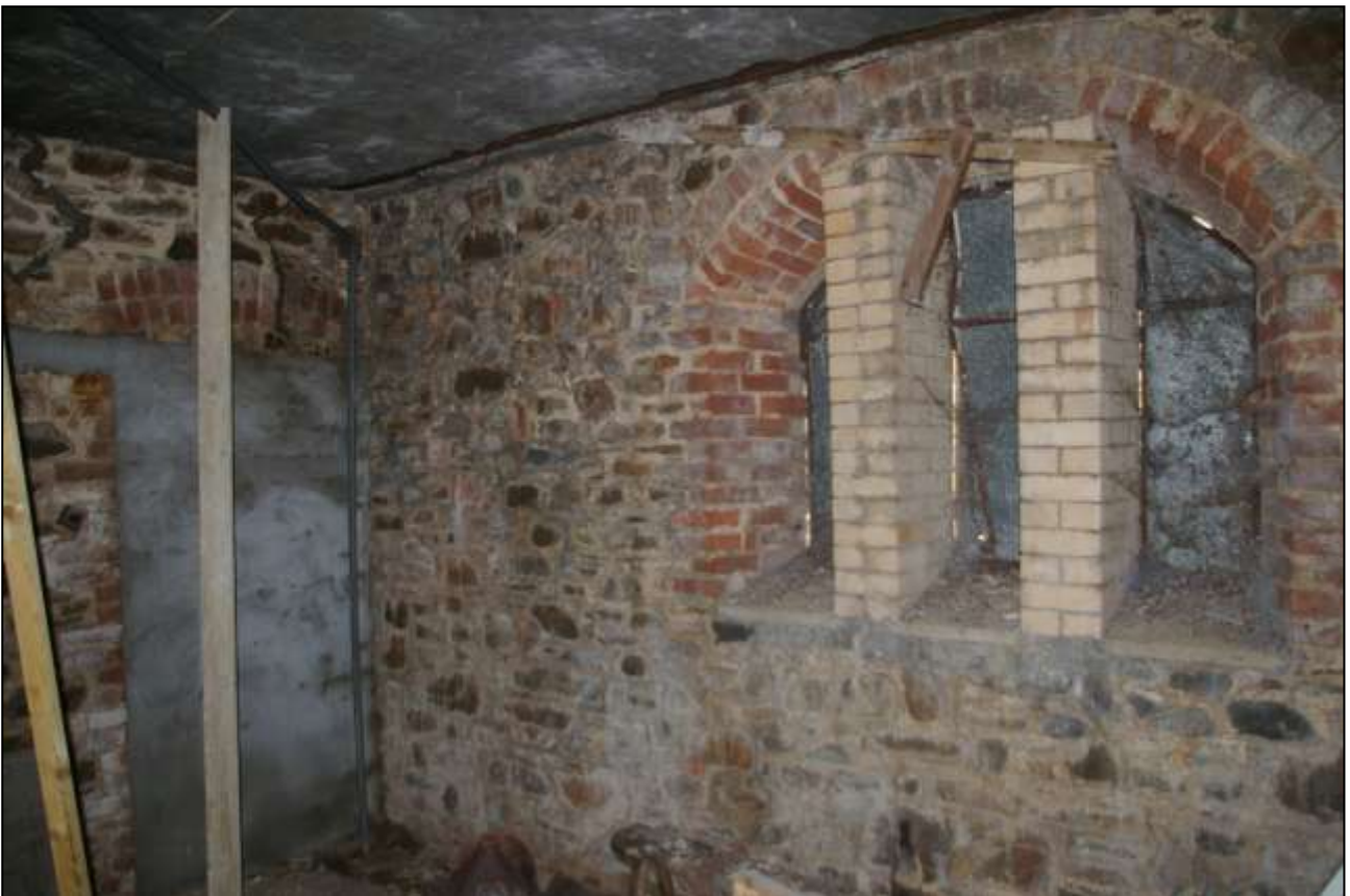
28. VIEW INSIDE THE BOILER ROOM, SHOWING WEST WINDOW, BLOCKED EXTERNALLY AND THE BLOCKED REAR DOORWAY; FROM THE NORTH-EAST.
