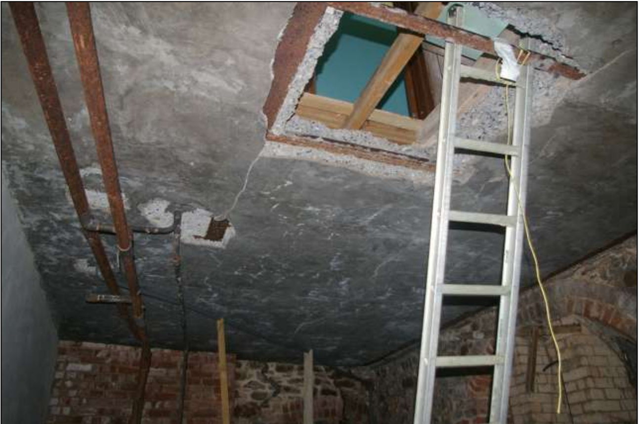
39. THE CONCRETE CEILING IN THE WESTERN END OF THE REAR CROSSWING, WHERE WOODEN JOISTS HAVE FAILED IN THE PAST, A LATER ALTERATION? FROM THE NORTH-EAST.
