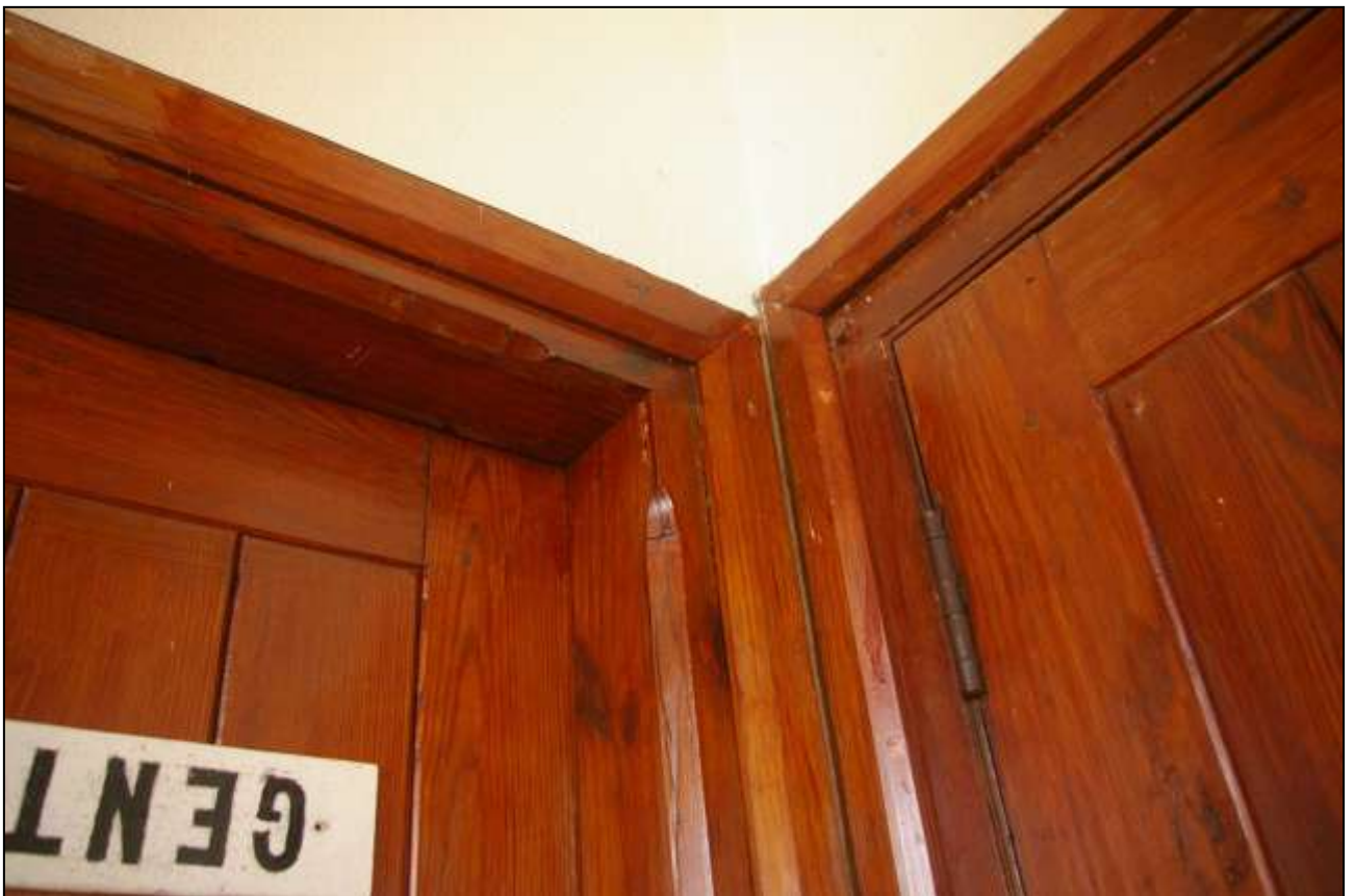
109. DETAILED VIEW OF THE DIFFERENT CHAMFERED OR BEADED DOORFRAMES IN THE BUILDING; FROM THE SOUTH-EAST.
