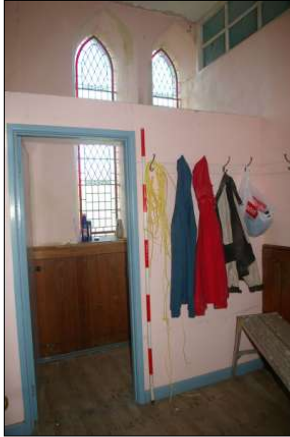
116. THE EVEN LATER PARTITION FORMING A LADIES TOILET CUBICLE; FROM THE SOUTH-EAST.
