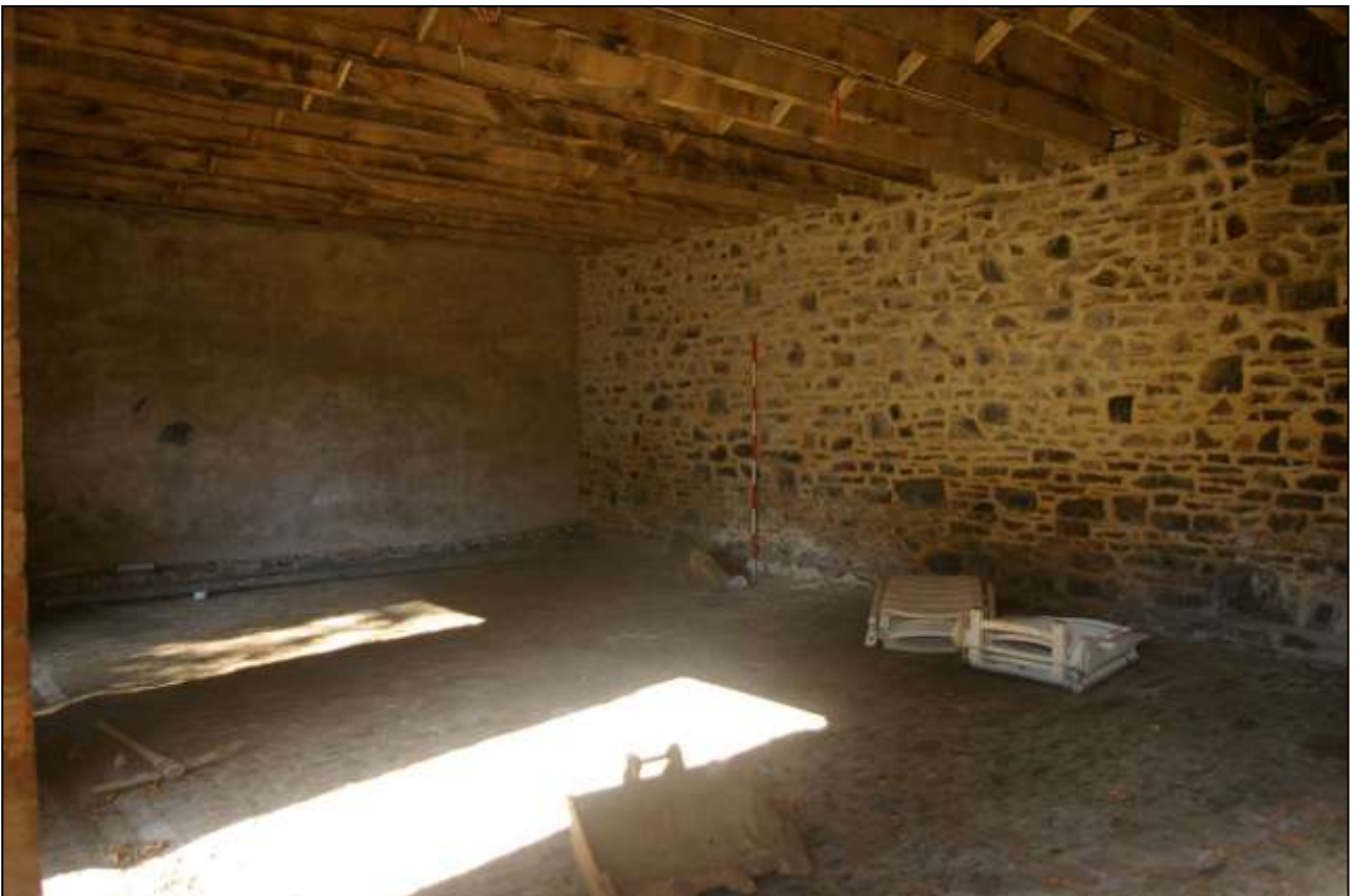
46. THE NORTH WALL OF THE CARRIAGE HOUSE AND THE INSERTED CONCRETE BLOCK PARTITION WALL; FROM THE SOUTH-EAST.
