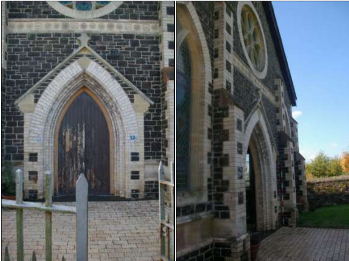
54. LEFT: THE FINE GOTHIC FRONT DOOR OF THE CHAPEL; FROM THE NORTH.
