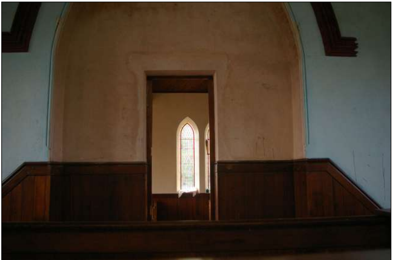
71. THE MODERN FORCING OF AN OPENING TO THE BACK OF THE ALCOVE ABOVE THE PULPIT; FROM THE NORTH.
