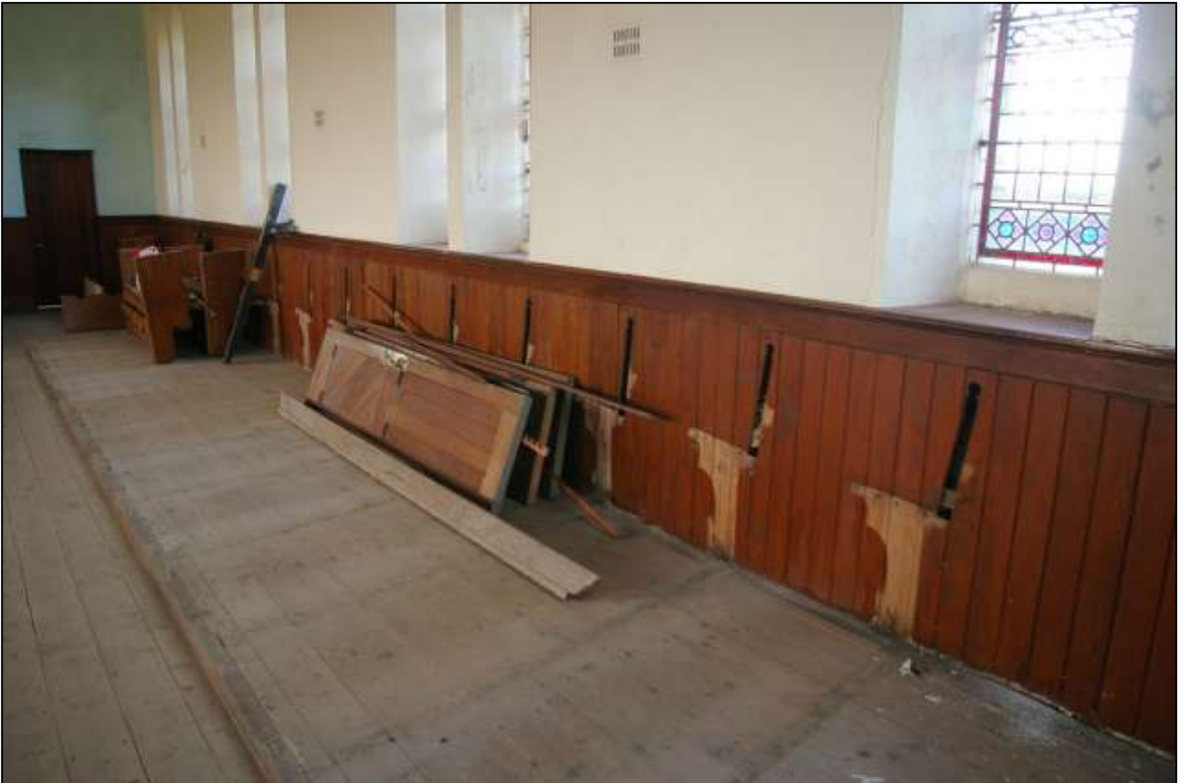
93. THE PANELLING TO THE WEST WALL, SHOWING THE SCARRING FROM THE REMOVED FITTED PEWS; FROM THE NORTH-NORTH-EAST.
