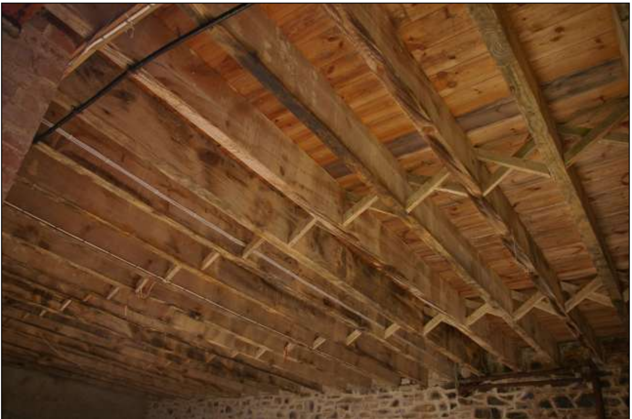
53. THE HEAVY JOISTS WHICH CARRY THE SUSPENDED FLOOR ABOVE WITH NOGGIN BRACES BETWEEN; FROM THE SOUTH-EAST.
