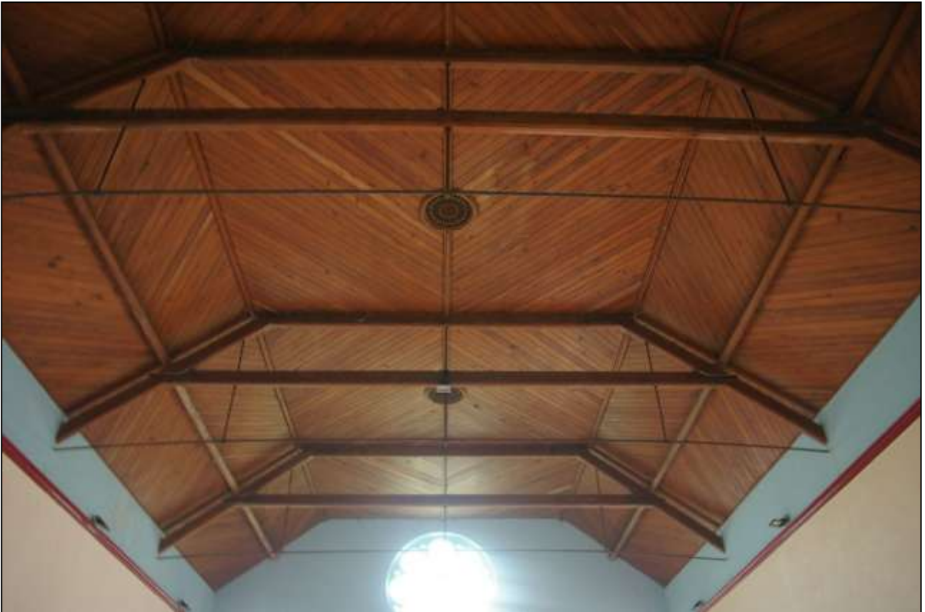
78. THE BOARDED ROOF IN THE CHAPEL; FROM THE SOUTH.
