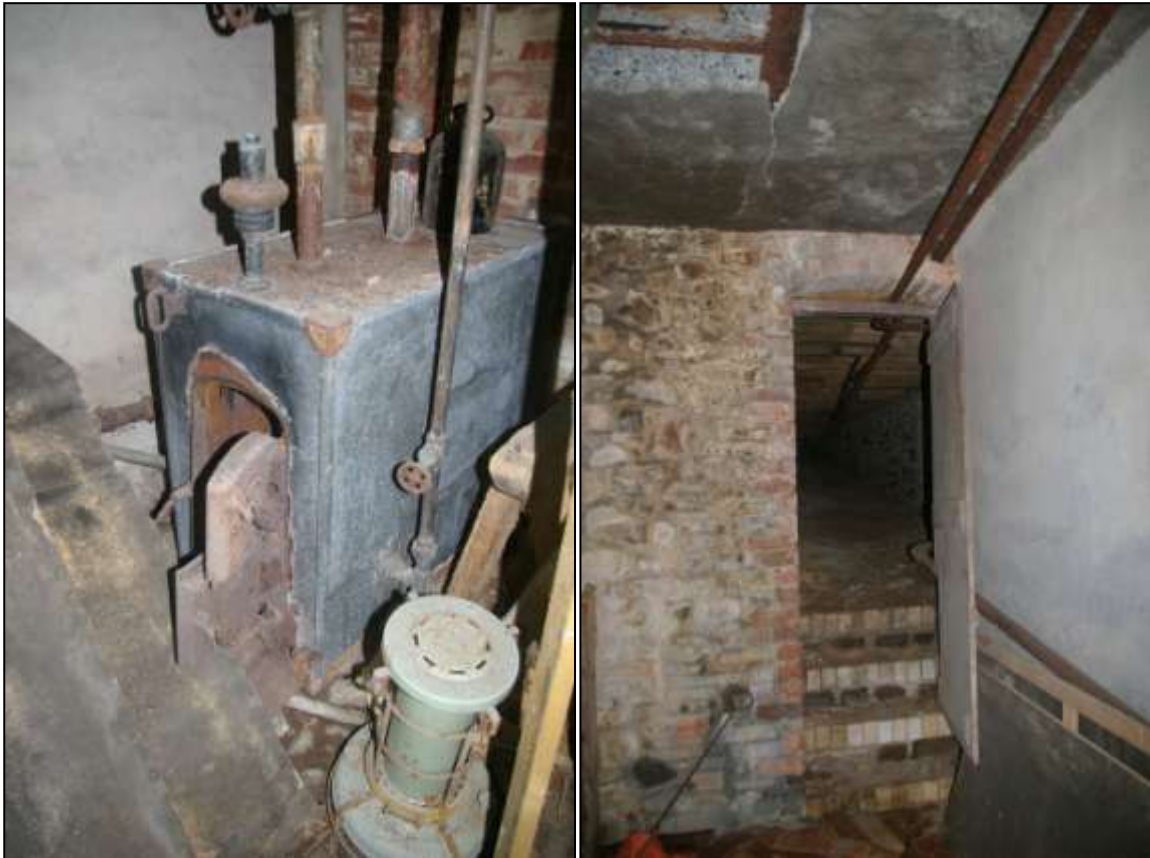
34. LEFT: THE BOILER; FROM THE NORTH-WEST.
