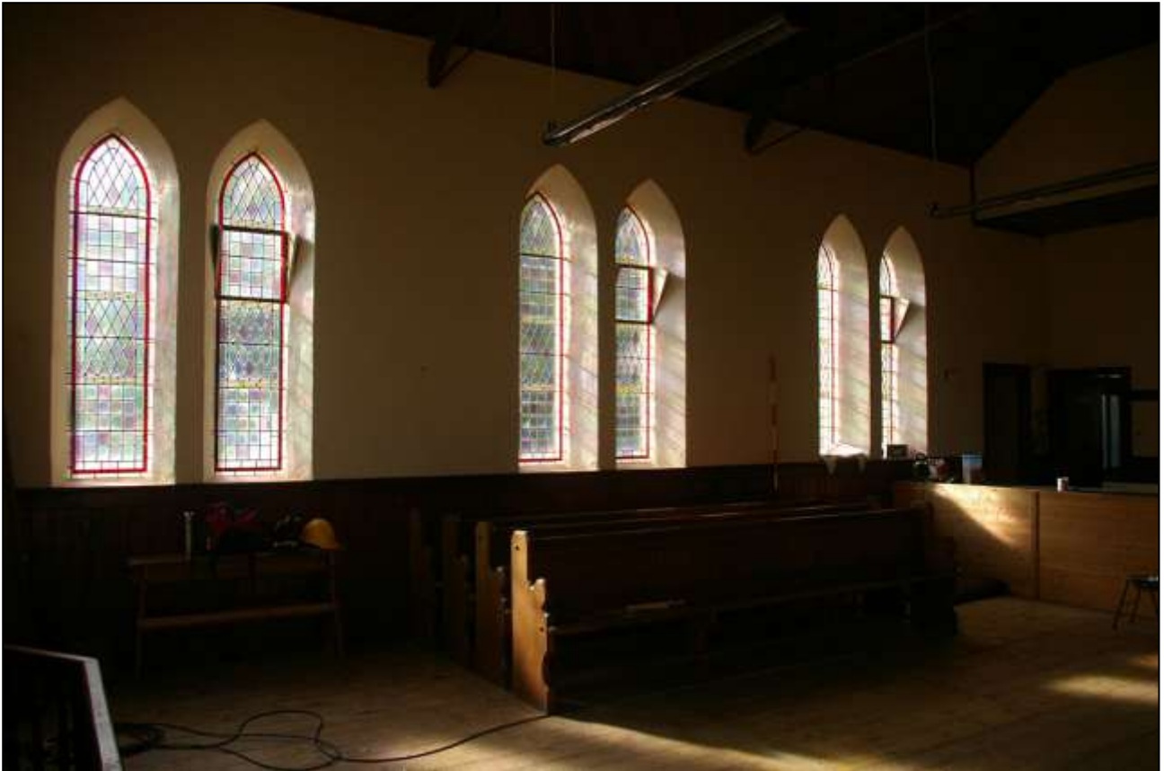
99. THE SOUTH WALL OF THE COMMUNITY HALL, WITH 2M SCALE; FROM THE NORTH-EAST.
