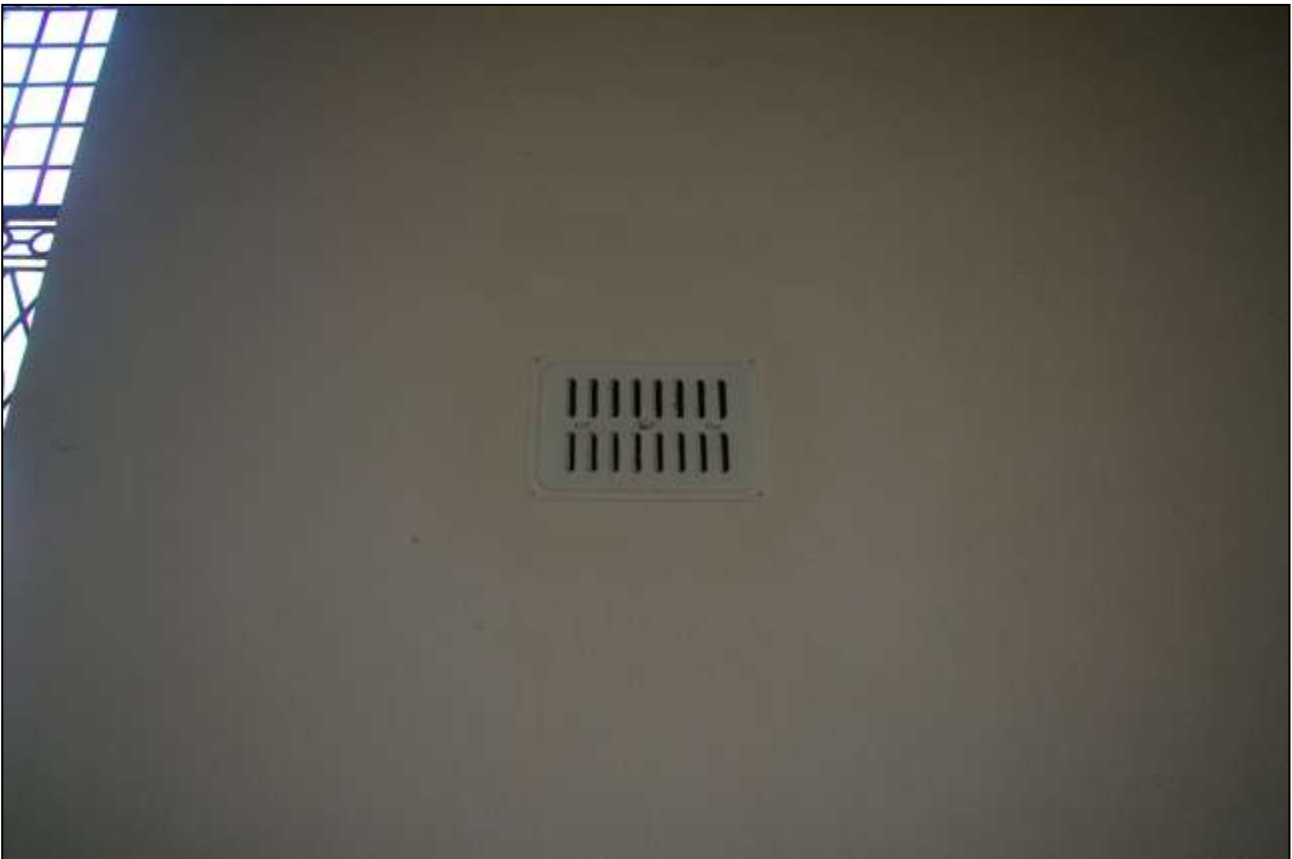
94. THE MORE MODERN METAL AIR VENT GRILLS ON THE WEST WALL; FROM THE NORTH-EAST.
