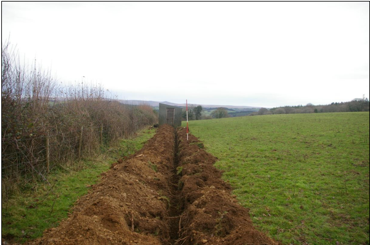
FIGURE 3: VIEW ALONG THE EAST-WEST ARM OF THE CABLE TRENCH; VIEWED FROM THE WEST (2M SCALE).
