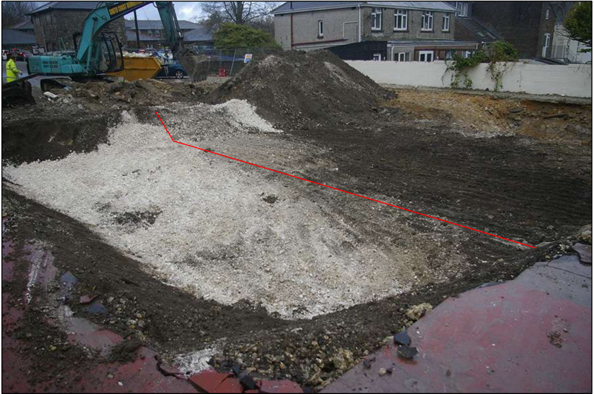
FIGURE 3: SITE SHOT MID REDUCTION OF LEVELS, THE APPROXIMATE LINE OF DEEPER TRUNCATION/FOOTING TO THE EASTERN TWO BAYS OF THE DEMOLISHED STRUCTURE IS SHOWN IN RED; VIEWED FROM THE SOUTH-WEST (NO SCALE).
