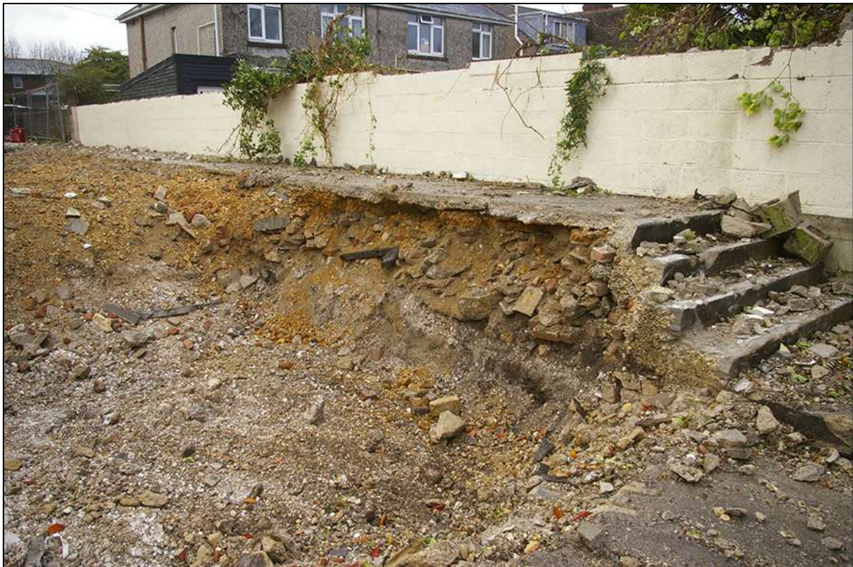
FIGURE 10: INSPECTION PIT IN SOUTH-EAST CORNER OF DEMOLISHED STRUCTURE; VIEWED FROM THE SOUTH-WEST (NO SCALE).
