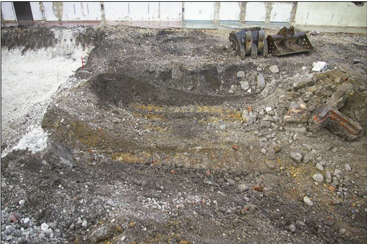
FIGURE 16: MADE-GROUND IN NORTH HALF OF SITE; BELOW THE DEPTH OF NATURAL IN THE SOUTH-WEST OF THE SITE DUE TO TRUNCATION AND IN-FILL; VIEWED FROM THE EAST (1M SCALE).
