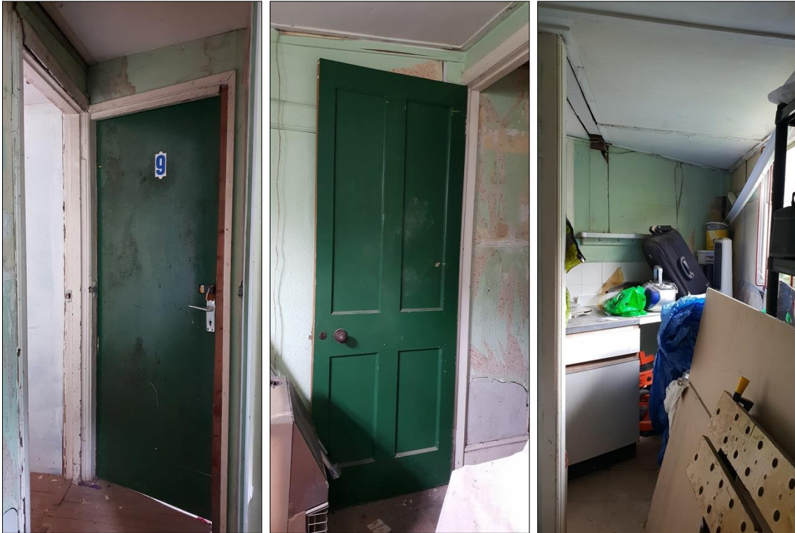
LEFT: DETAIL SOUTHERN OF THE INTERNAL DOORS WITHIN B1.2; VIEWED FROM THE SOUTH.
