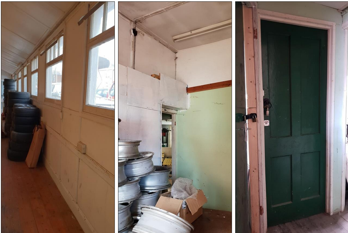
LEFT: DETAIL OF THE INTERNAL NORTH-EAST ELEVATION OF THE MAIN ROOM OF B1.1; VIEWED FROM THE SOUTH-EAST.
