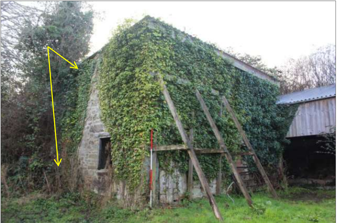
THE NORTH AND EAST ELEVATIONS OF FB1; VIEWED FROM THE NORTH-EAST (SCALE 2M). THE EXTERNAL BUTTRESS IS INDICATED.
