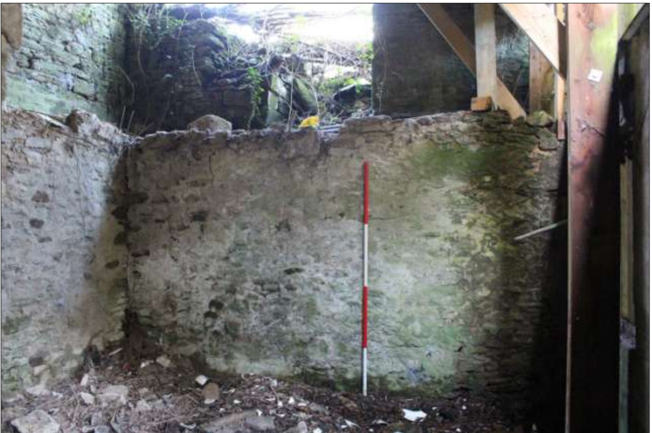
THE GF NORTH WALL OF FB2B; VIEWED FROM THE SOUTH (SCALE 2M).
