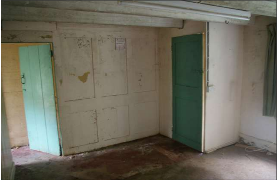
FIGURE 12: THE 18 TH CENTURY PARTITION WALL BETWEEN R1 AND R2, FROM R1; VIEWED FROM THE SOUTH-WEST (NO SCALE).
