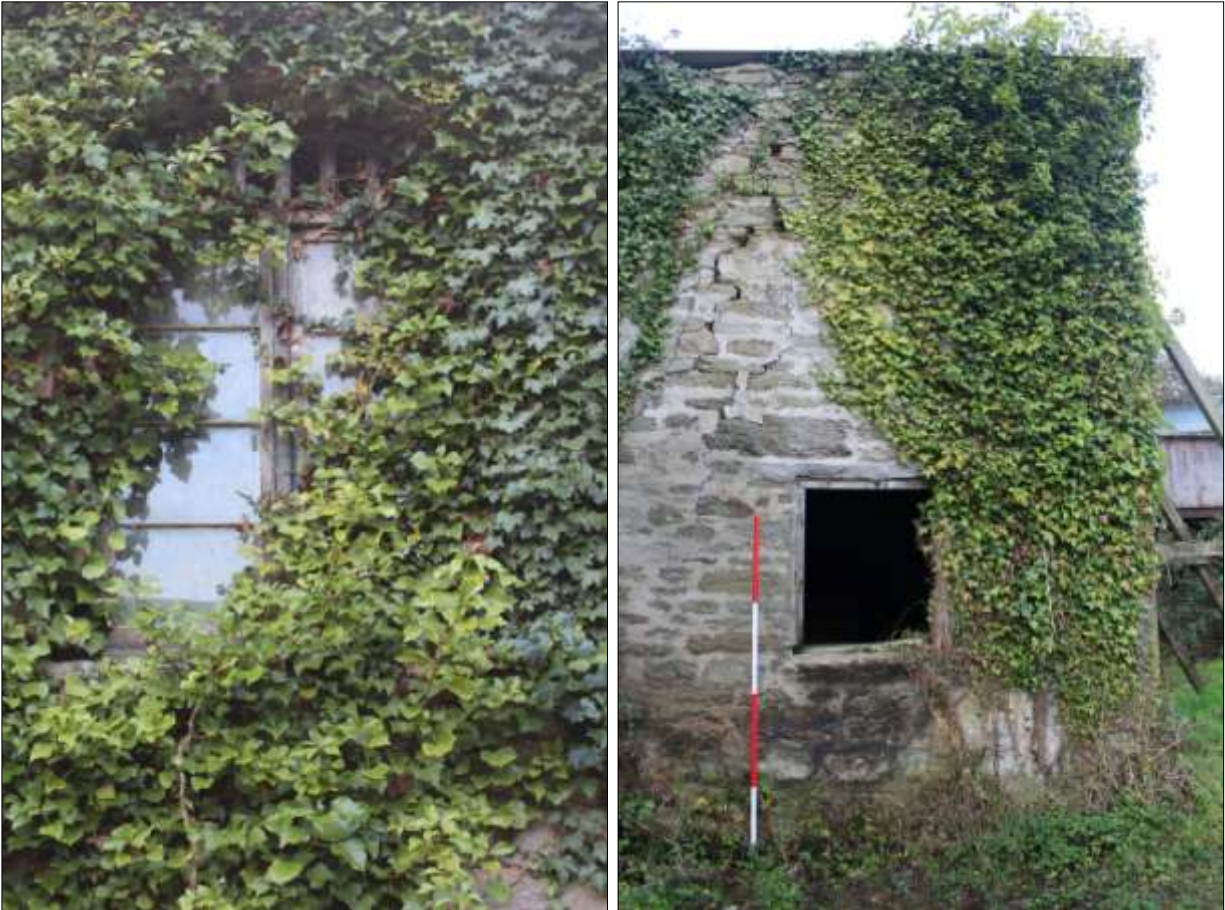
LEFT: D9 IN THE NORTH ELEVATION OF FB1 AT FF LEVEL; VIEWED FROM THE NORTH. RIGHT: THE EAST ELEVATION OF FB1, SHOWING W1; VIEWED FROM THE EAST (SCALE 2M).
