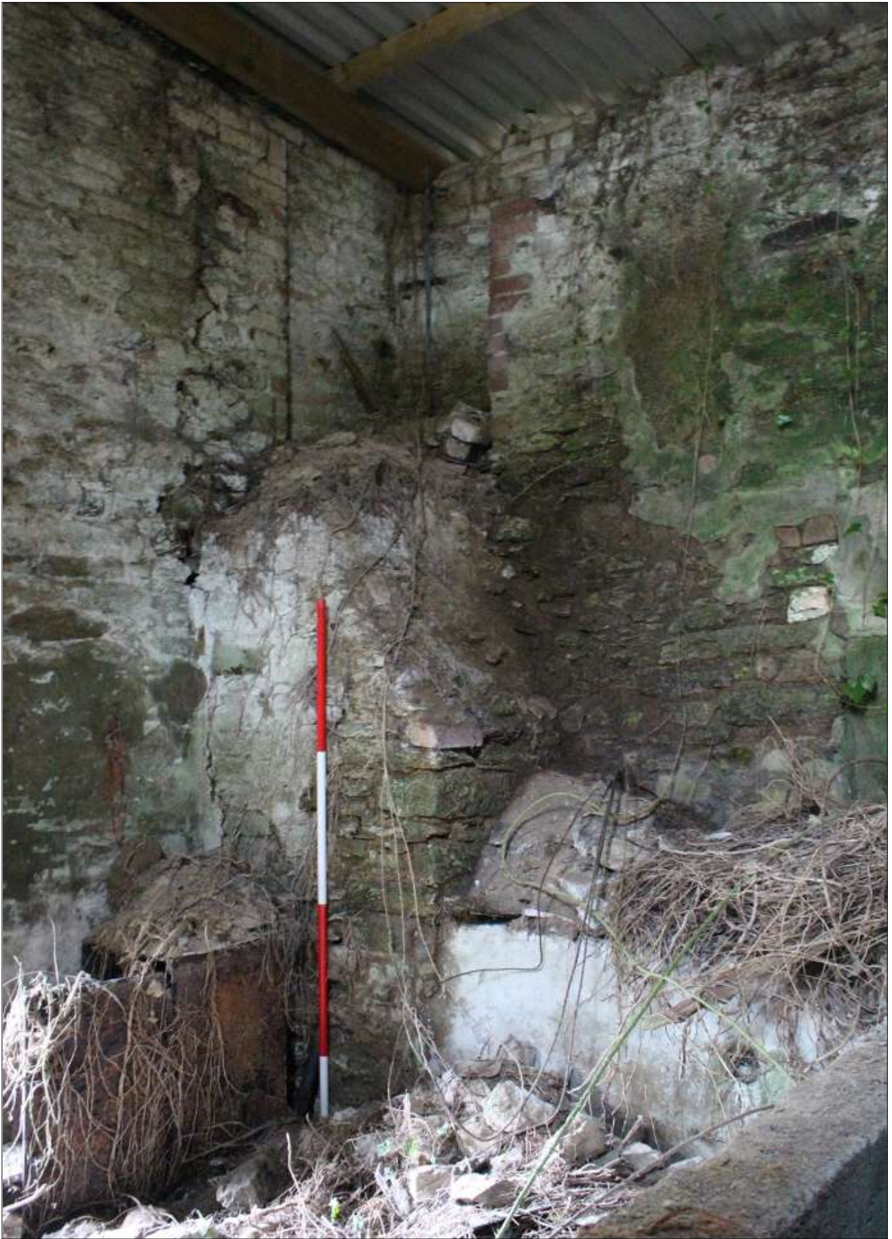
THE INTERNAL SOUTH-EAST CORNER OF FB1 SHOWING THE BLOCK OF MASONRY (BOILER/OVEN?); VIEWED FROM THE NORTH-WEST (SCALE 2M).
