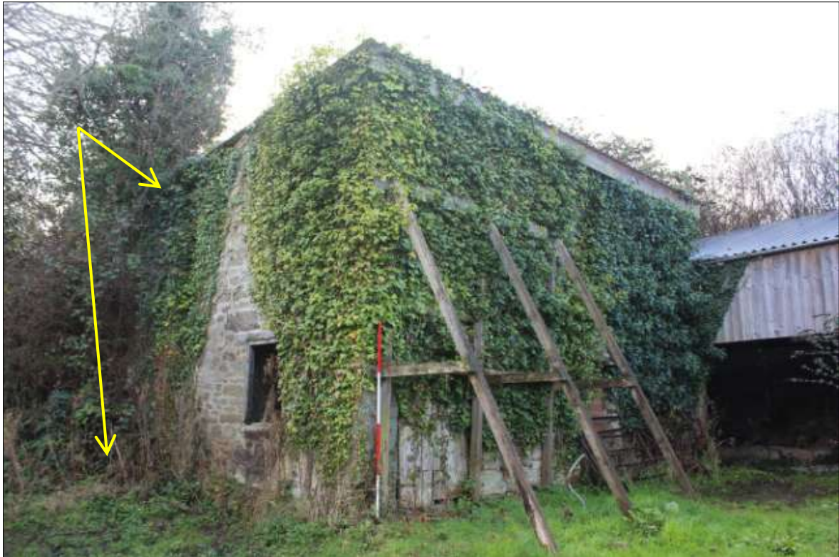
FIGURE 20: THE NORTH AND EAST ELEVATIONS OF FB1; VIEWED FROM THE NORTH-EAST (SCALE 2M). THE EXTERNAL BUTTRESS IS INDICATED.
