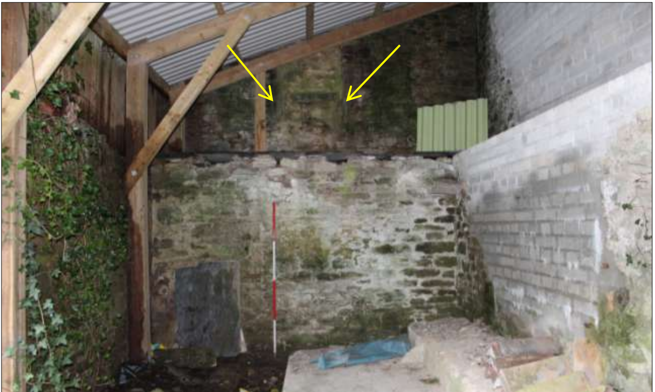
THE SOUTH END OF FB2A, BO2 IS INDICATED; VIEWED FROM THE NORTH (SCALE 2M).
