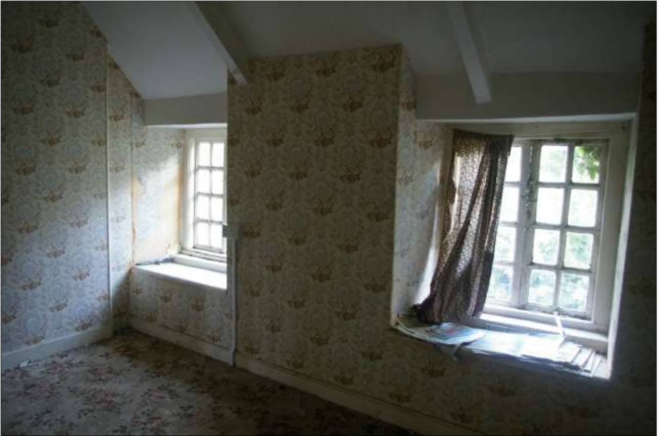
THE EAST WALL OF R8 WITH WF2 AND WF3; VIEWED FROM THE SOUTH-WEST.
