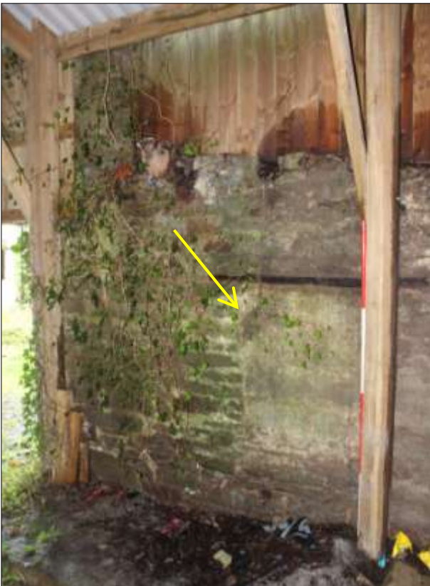
THE SHARED WALL BETWEEN FB1 AND FB2A, SHOWING BO1 (INDICATED); VIEWED FROM THE SOUTH-WEST (SCALE 2M).
