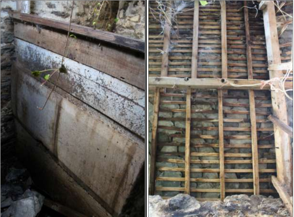
LEFT: THE REUSED RAISED AND FIELDED PANELS IN FB4B; VIEWED FROM THE SOUTH-EAST. RIGHT: THE ROOF OF FB4B; VIEWED FROM BENEATH.
