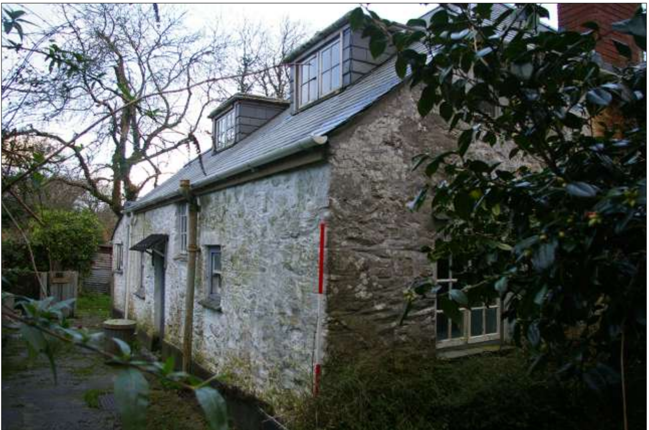
THE WEST AND SOUTH ELEVATIONS OF THE COTTAGE; VIEWED FROM THE SOUTH-WEST (SCALE 2M).
