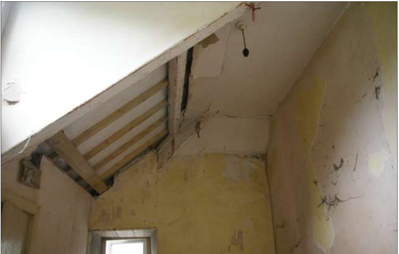
THE CEILING IN R9 SHOWING THE C21 REPLACEMENT ROOF ELEMENTS; VIEWED FROM THE SOUTH.
