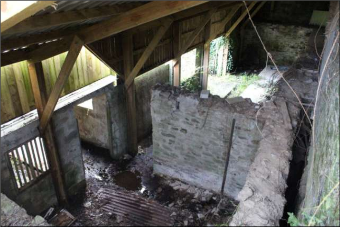
THE INTERIOR OF B2, LOOKING DOWN INTO THE STRUCTURE; VIEWED FROM THE NORTH.
