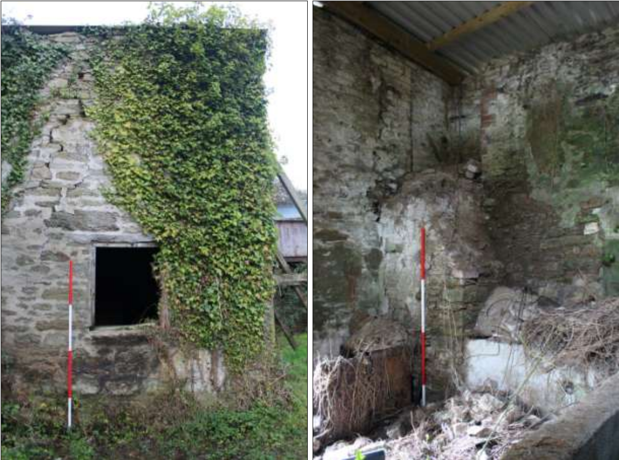
LEFT FIGURE 21: THE EAST ELEVATION OF FB1; VIEWED FROM THE EAST (SCALE 2M).
