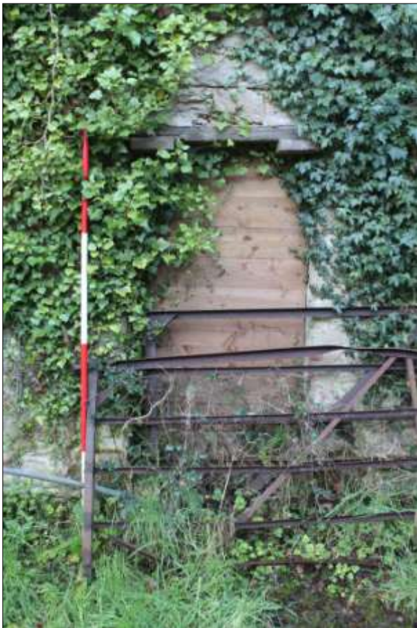
LEFT: FORCED DOORWAY D2; VIEWED FROM THE NORTH (SCALE 2M).
