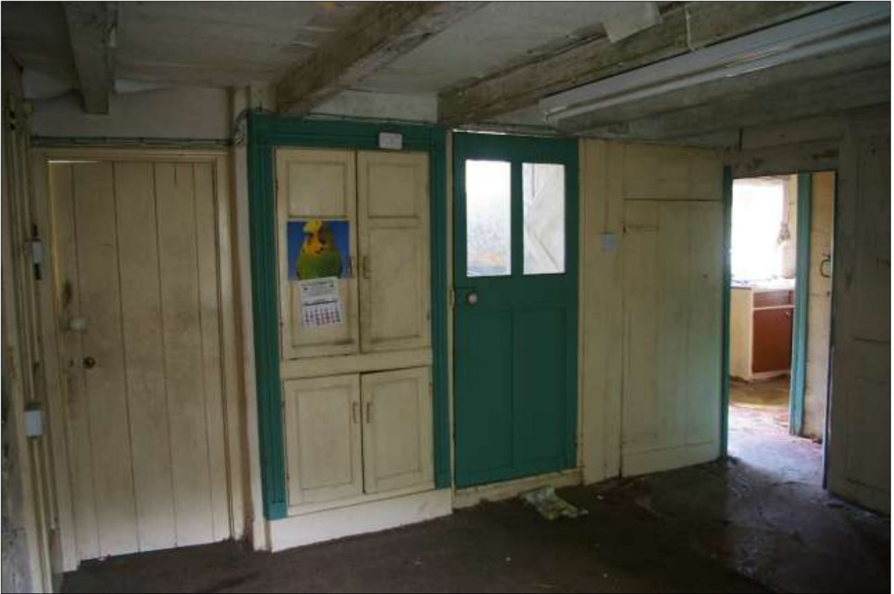
THE WEST WALL OF R1, WITH DOORS TO R4 (LEFT), THE STAIRS (CENTRE) AND R3 (RIGHT); VIEWED FROM THE SOUTH-EAST.
