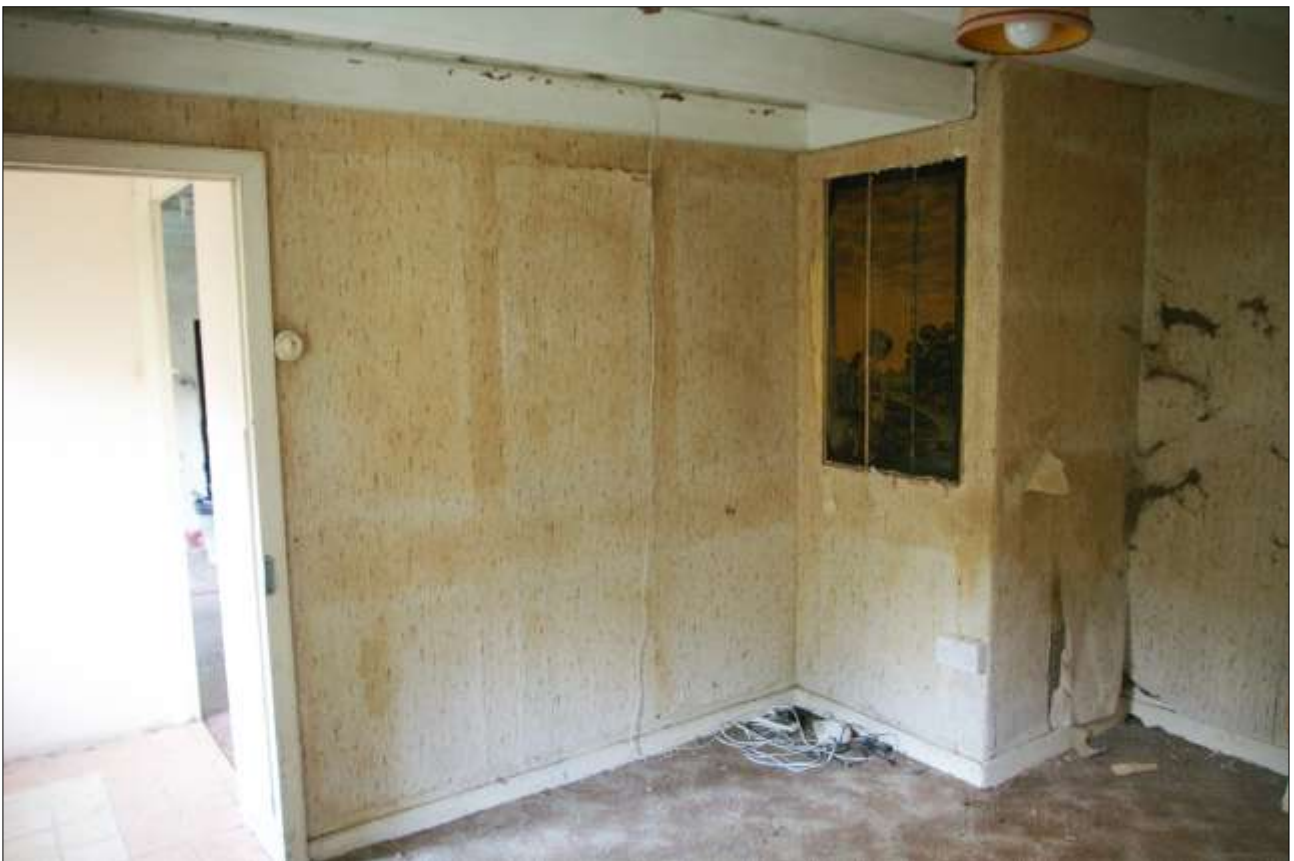
THE 18 TH CENTURY PARTITION WALL BETWEEN R1 AND R2, FROM R2; VIEWED FROM THE NORTH-EAST (NO SCALE). THE COVERED PANELS ARE VISIBLE, WITH THE EXPOSED PANEL TO THE RIGHT.
