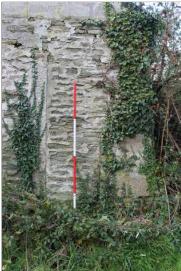
AS ABOVE, DETAIL OF THE NORTH-EAST CORNER AND GRANITE POST; VIEWED FROM THE EAST (SCALE 2M).
