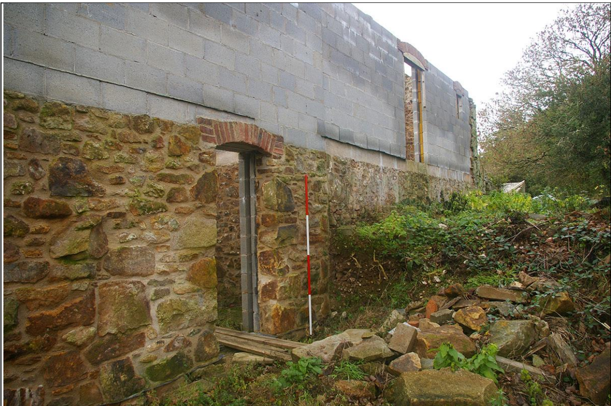
THE REAR DOOR IN THE NORTH ELEVATION OF BUILDING 2 AND THE CLEAR BUILD LINE TO BUILDING 1, WITH THE ATTACHED/ADJACENT WHIM MOUND; FROM THE NORTH-EAST.
