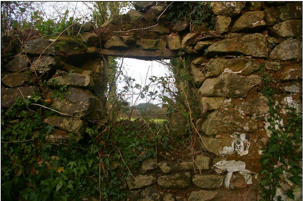
FIGURE 8: THE WINDOW IN BUILDING 3, WITH WEATHERED TIMBER LINTEL; FROM THE SOUTH.
