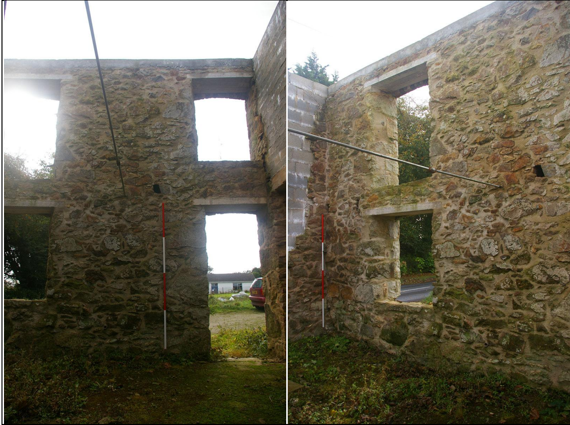
LEFT: THE INNER FACE OF THE SOUTH WALL OF BUILDING 2 AND ITS UNCOMFORTABLE RELATIONSHIP WITH BUILDING 1; FROM THE NORTH. RIGHT: AS ABOVE, SHOWING THE APPARENT REBUILDING AROUND THE 'WINDOW' OPENINGS; FROM THE NORTH-WEST.
