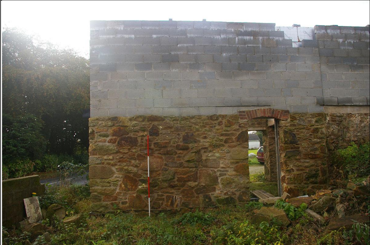
THE NORTH ELEVATION OF BUILDING 2, SHOWING IT HAS BEEN TOTALLY REBUILT DUE TO THE INTEGRAL DAMP COURSE; FROM THE NORTH.
