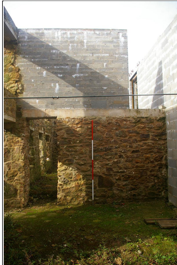
THE PARTITION WALL TO BUILDING 1, REBUILT OR HEAVILY REPOINTED STONE BELOW AND CONCRETE BLOCK ABOVE; FROM THE EAST.
