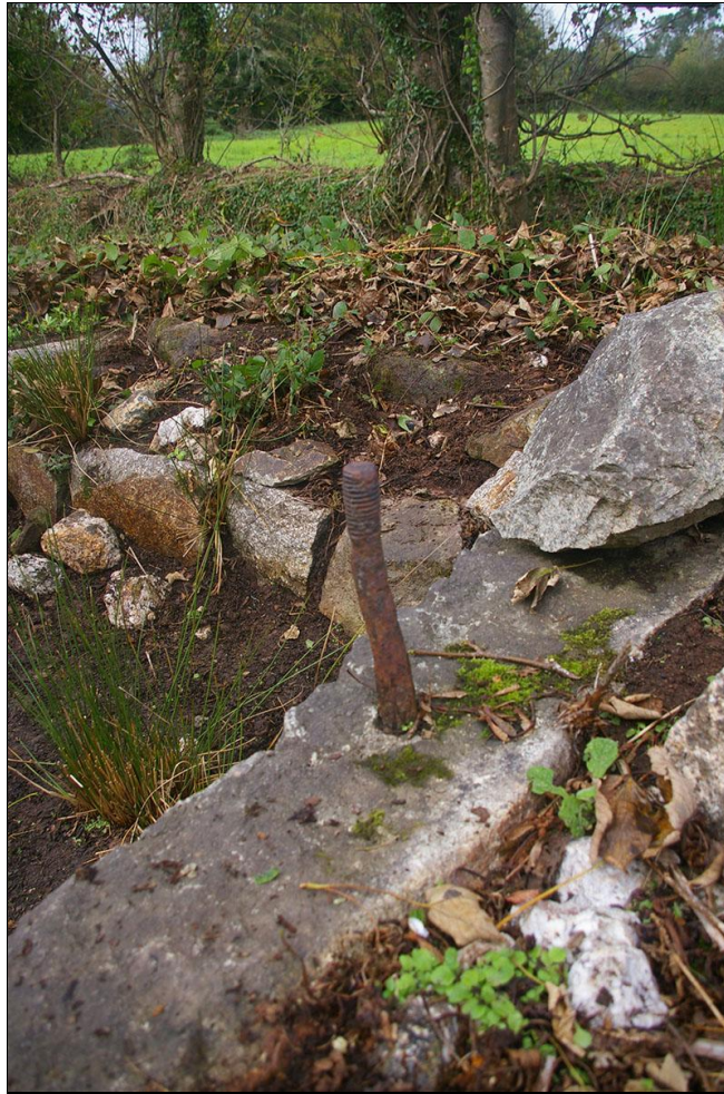
METAL FIXING WITH CORRODED SCREW THREAD, SET IN THE GRANITE POST TO THE EAST SIDE; FROM THE SOUTH-EAST.
