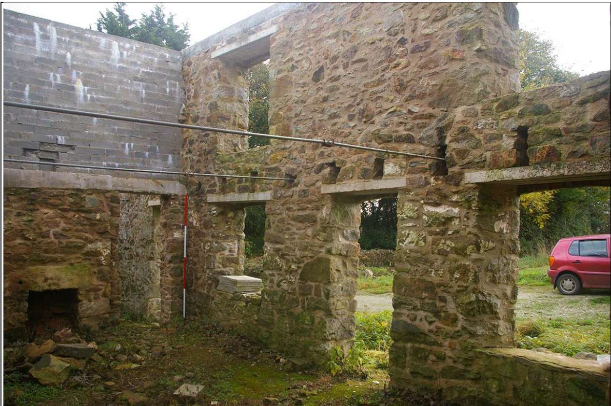
THE SOUTH AND EAST WALLS OF BUILDING 1, SHOWING THE DOOR THROUGH TO BUILDING 2 AND THE FIREPLACE AND STACK ON THE EAST WALL; FROM THE NORTH-WEST.
