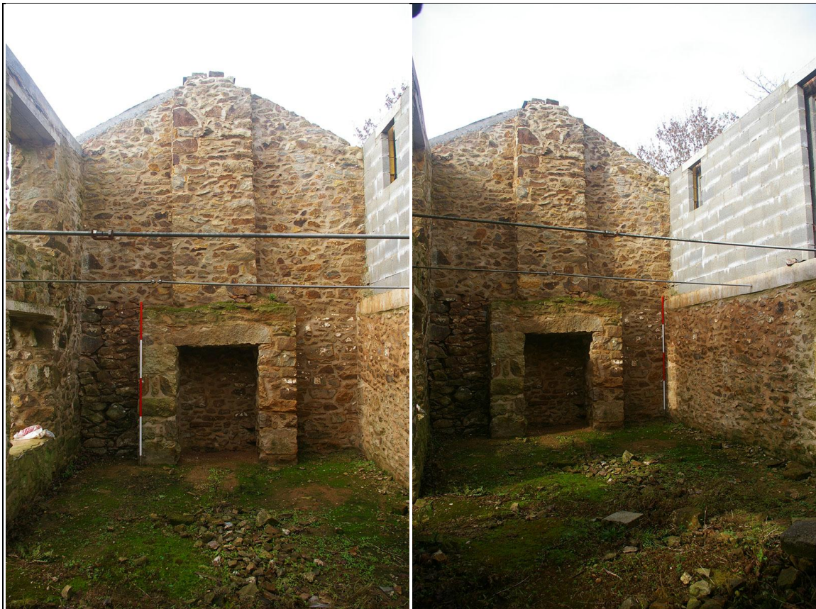
LEFT: THE INNER FACE OF THE WEST GABLE OF BUILDING 1, SHOWING REBUILT STACK AND THE POSSIBLE OPEN HEARTH; FROM THE EAST. RIGHT: THE WEST AND NORTH WALLS OF BUILDING 1, SHOWING THE CHANGES IN CHARACTER TO BUILD ON BOTH WALLS; FROM THE SOUTH-EAST.
