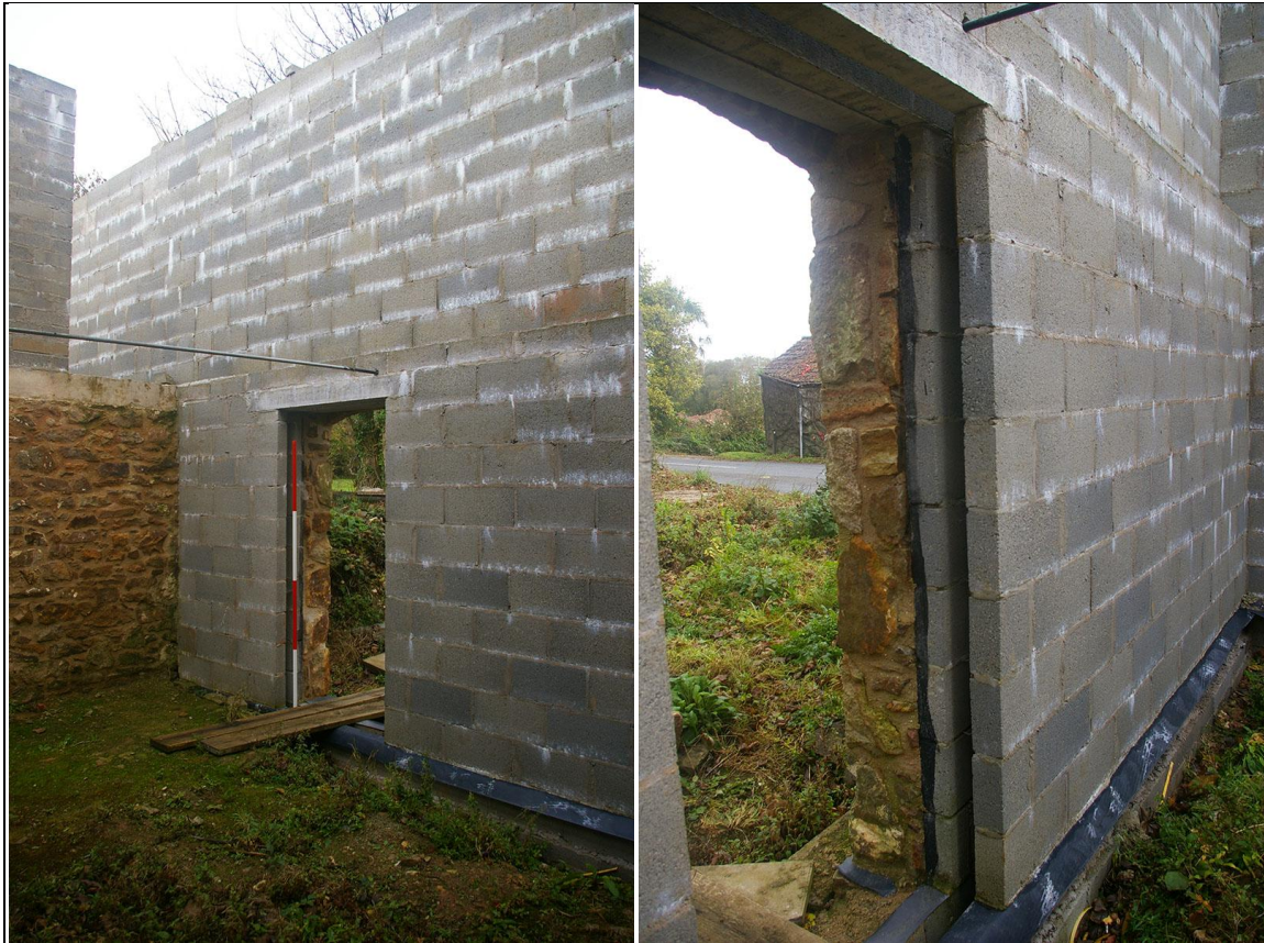
LEFT: THE NORTH WALL OF BUILDING 2, WITH THE REAR DOOR AND PARTITION WALL TO BUILDING 1; FROM THE SOUTH-EAST. RIGHT: DETAIL OF THE MODERN CONCRETE BLOCK CAVITY WALL CONSTRUCTION IN BUILDING 2; FROM THE WEST, SOUTH-WEST.
