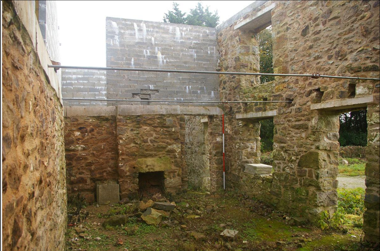
THE EAST WALL, SHOWING THE VERY DIFFERENT CHARACTER OF THE STONEMWORK FROM THE SOUTH AND EVEN NORTH OR WEST WALLS, ALSO HEAVY REPOINTING IN CEMENT AND CONCRETE RING BEAM AND BLOCKS ABOVE; FROM THE NORTH-WEST.
