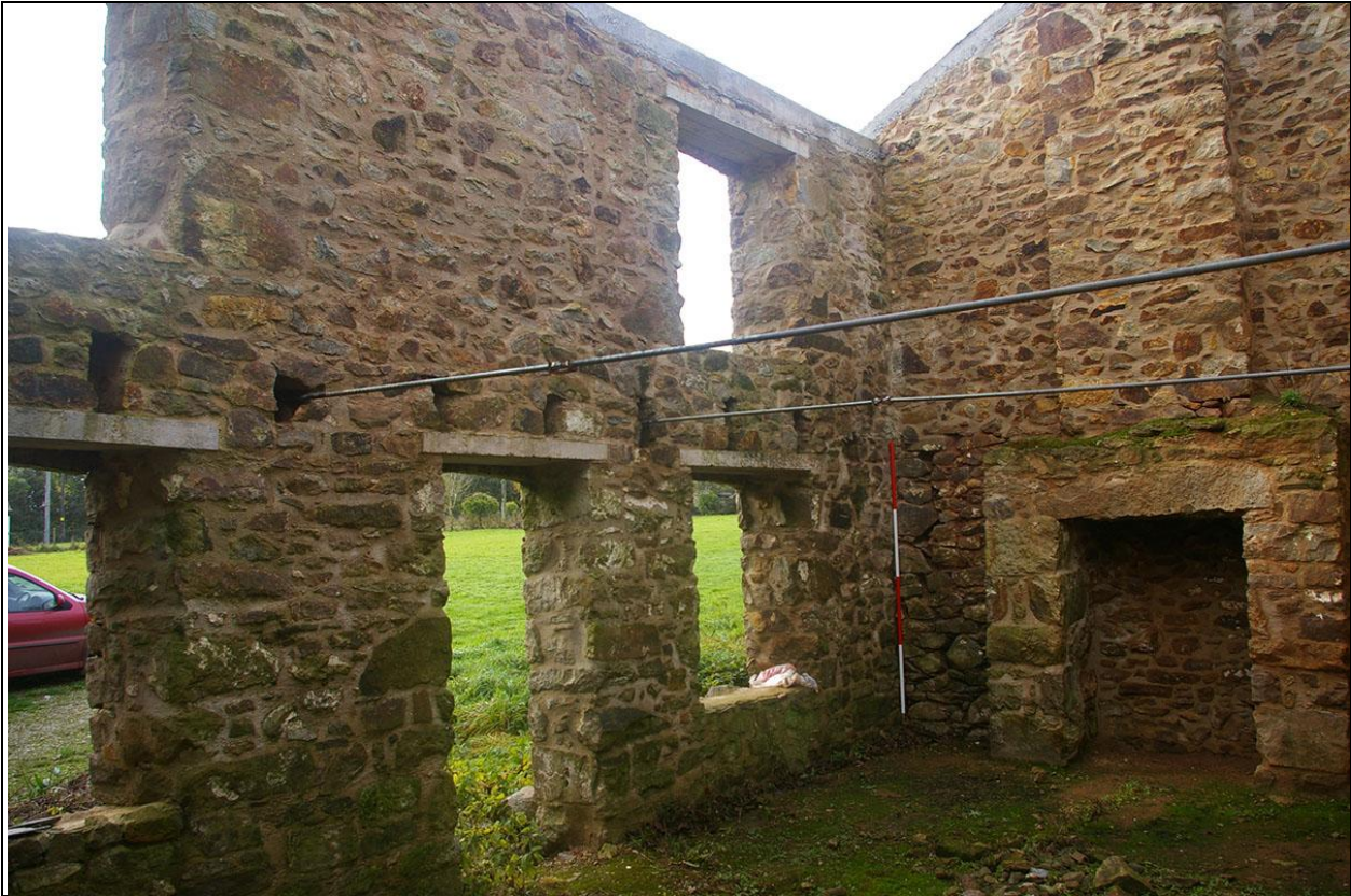
THE WEST AND SOUTH WALLS OF BUILDING 1, SHOWING A SIMILAR CHANGE IN CHARACTER AT APPROX 2M HEIGHT, BELOW HEAVIER IRREGULAR BUILD, GREEN MOSSY STONES, REPOINTED, ABOVE LOOKING REBUILT; FROM THE NORTH-EAST.
