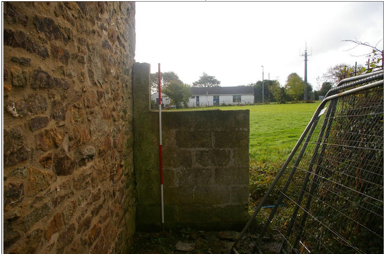
THE REPLACED FRONT WALL OF BUILDING 3, OR INFILLED OPENING, USING CONCRETE BLOCKS; FROM THE NORTH.
