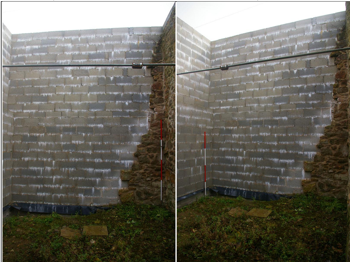
LEFT: THE EAST WALL OF BUILDING 2, TOTALLY REPLACED IN CONCRETE BLOCK; FROM THE WEST. RIGHT: THE EAST AND NORTH WALLS OF BUILDING 2, BOTH REBUILT, TO THE EAST IN CONCRETE BLOCK, TO THE NORTH CONCRETE BLOCK CLAD IN STONE RUBBLE; FROM THE SOUTH-WEST.
