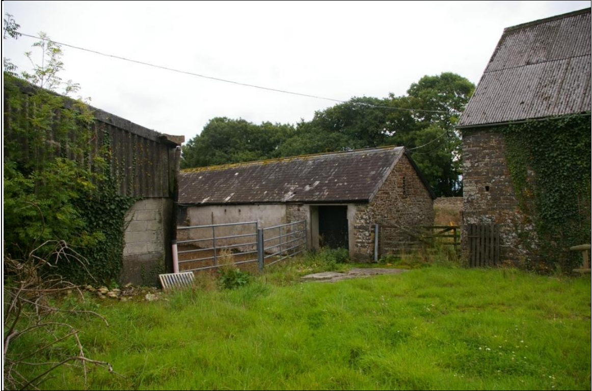
19. THE NORTH ELEVATION OF THE NORTH RANGE OF THE 19 TH CENTURY FARMYARD WHICH WILL BE ABUTTED AND SCREENED BY THE PROPOSALS; FROM THE NORTH-WEST.
