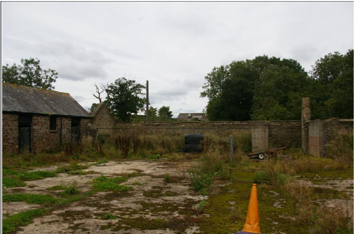
14. VIEW OF THE RUINED EASTERN BUILDING IN THE 19 TH CENTURY FARMYARD AND VIEWS OVER ITS RUINS TO THE OUTBARN; FROM THE SOUTH-WEST.
