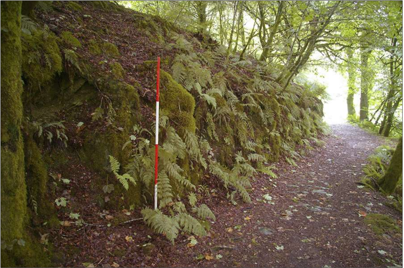
39. PATHWAY FROM SIMONSBATH HOUSE LEADING TO ASHCOMBE GARDEN, JUST SOUTH OF THE GARDEN, SHOWING NATURAL ROCK BEHIND THE REVETMENT FACE; VIEWED FROM THE SOUTH-SOUTH-WEST (2M SCALE).
