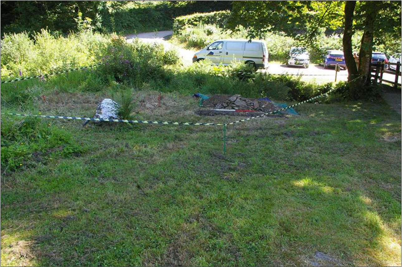
18. TRENCHES 3 AND 4 IN RELATION TO THE EXISTING FOOTBRIDGE; VIEWED FROM THE WEST (1M SCALE).
