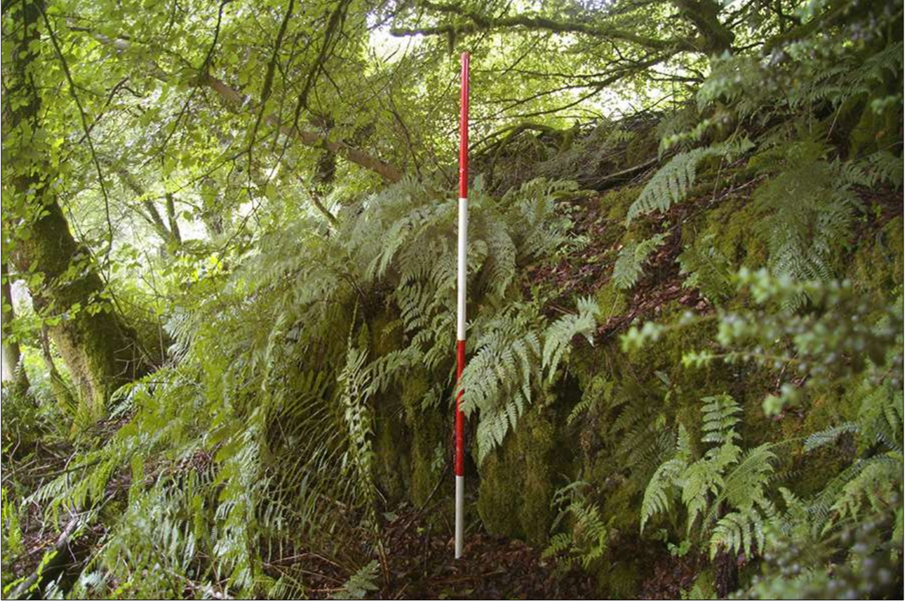
35. BOUNDARY WALL ADJACENT TO PUBLIC TOILETS AND NORTH-WEST OF ASHCOMBE COTTAGE; VIEWED FROM THE SOUTH (2M SCALE).
