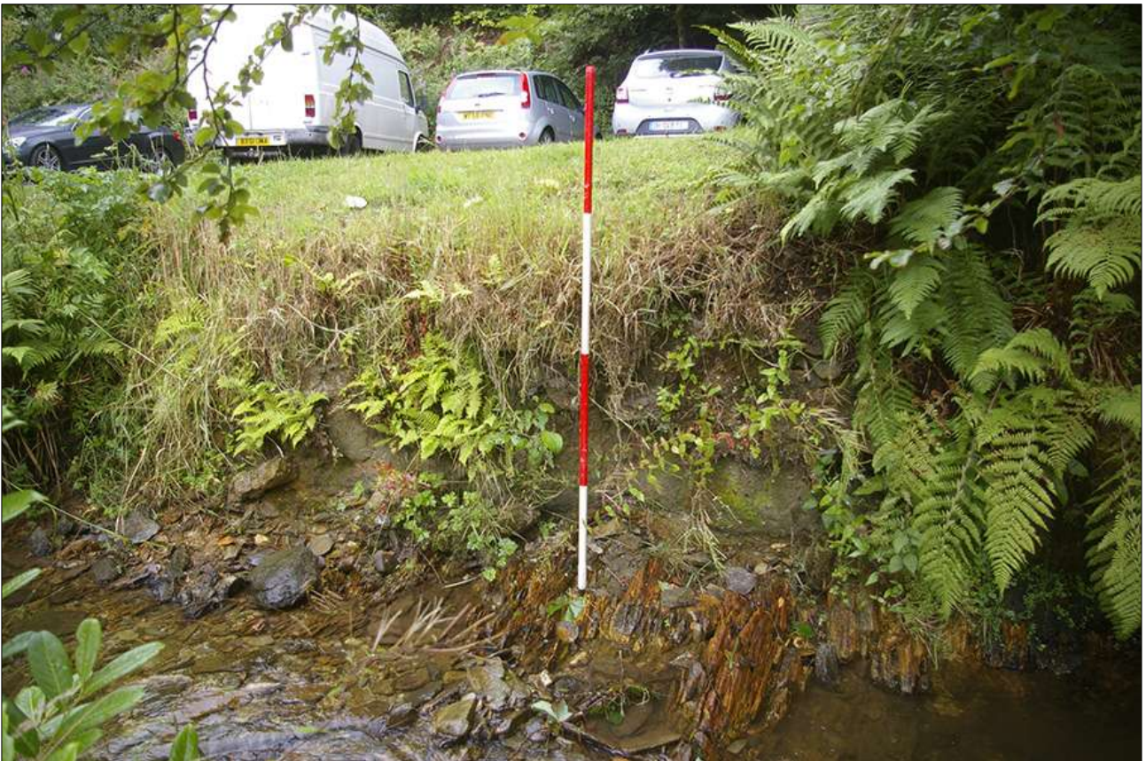
36. RIVER BANK ADJACENT TO ASHCOMBE CAR PARK; VIEWED FROM THE WEST (2M SCALE).
