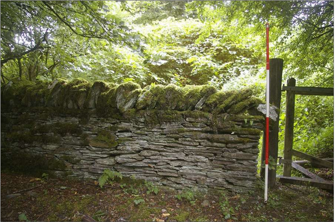
41. EXAMPLE SECTION OF DEFINITIVE BOUNDARY WALLS TO THE FIELDS NORTH-WEST OF THE SITE AND IN THE AREA OF SIMONSBATH; VIEWED FROM THE SOUTH (2M SCALE).
