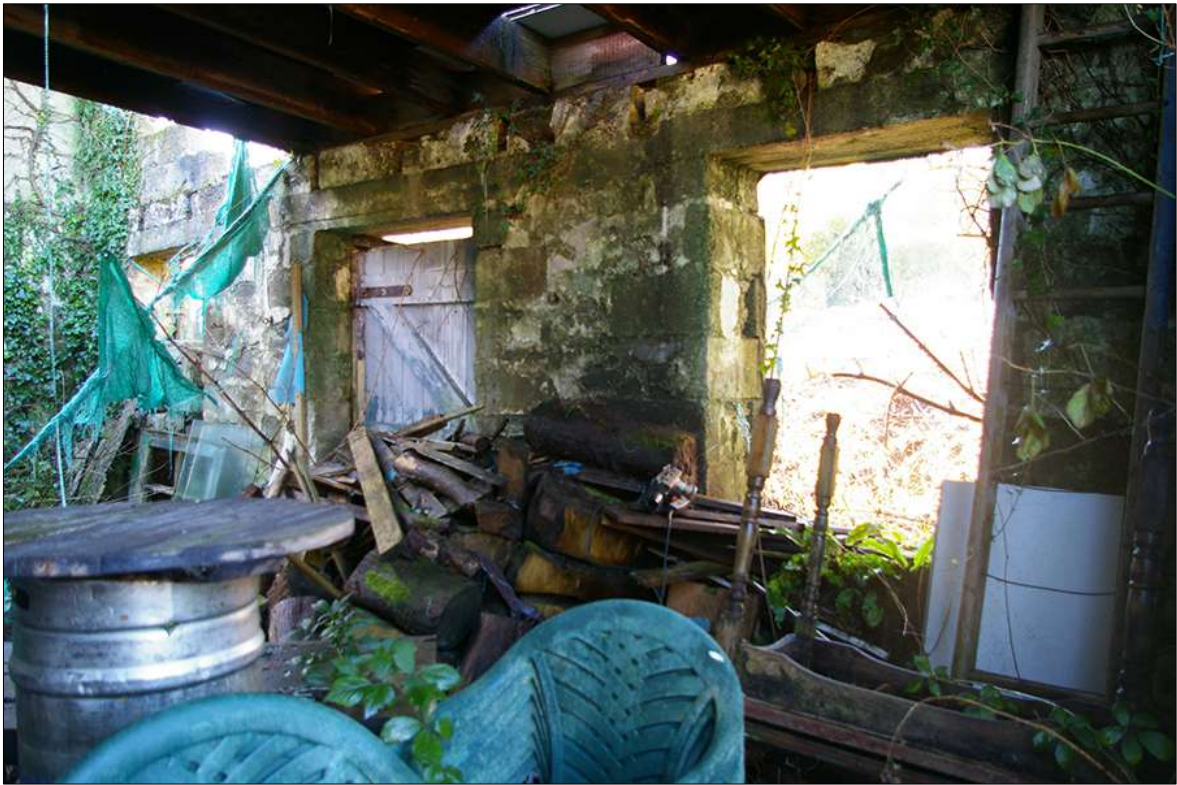
PHOTO 7: DETAIL OF THE INTERNAL WEST ELEVATION OF THE DERELICT OUTBUILDING WITHIN FIELD 1; FACING SOUTH-WEST.
