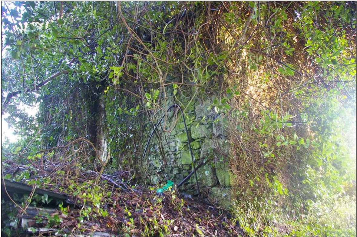
FIGURE 10: VIEW OF THE DERELICT BUILDING IN THE SOUTH-EAST CORNER OF FIELD 2; FACING NORTH-EAST.
