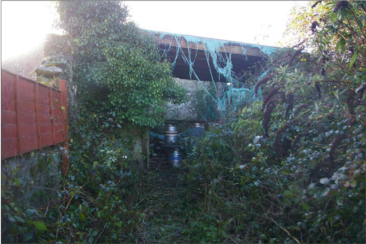
PHOTO 5: DETAIL OF THE DERELICT OUTBUILDING TO THE REAR OF THE PACKHORSE INN, SOUTH-EAST CORNER OF FIELD 1; FACING SOUTH.
