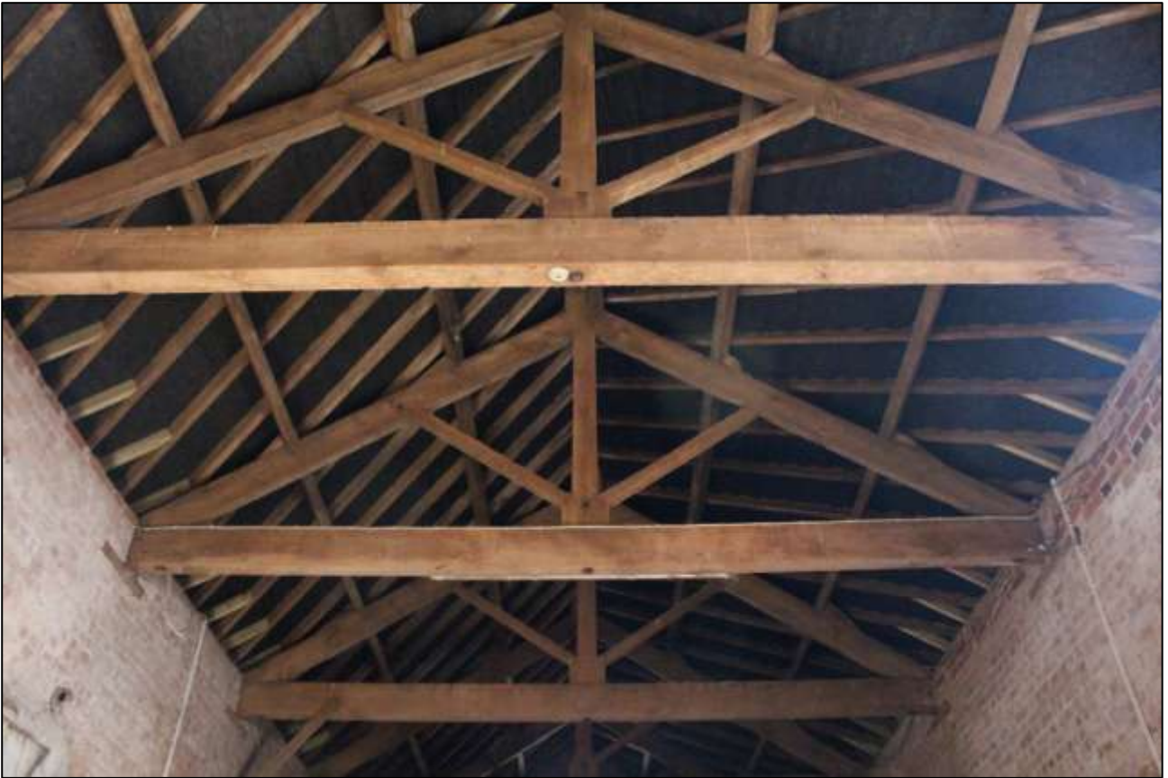
B6 FF INTERIOR, DETAIL OF THE FINE KINGPOST ROOF; VIEWED FROM THE SOUTH.
