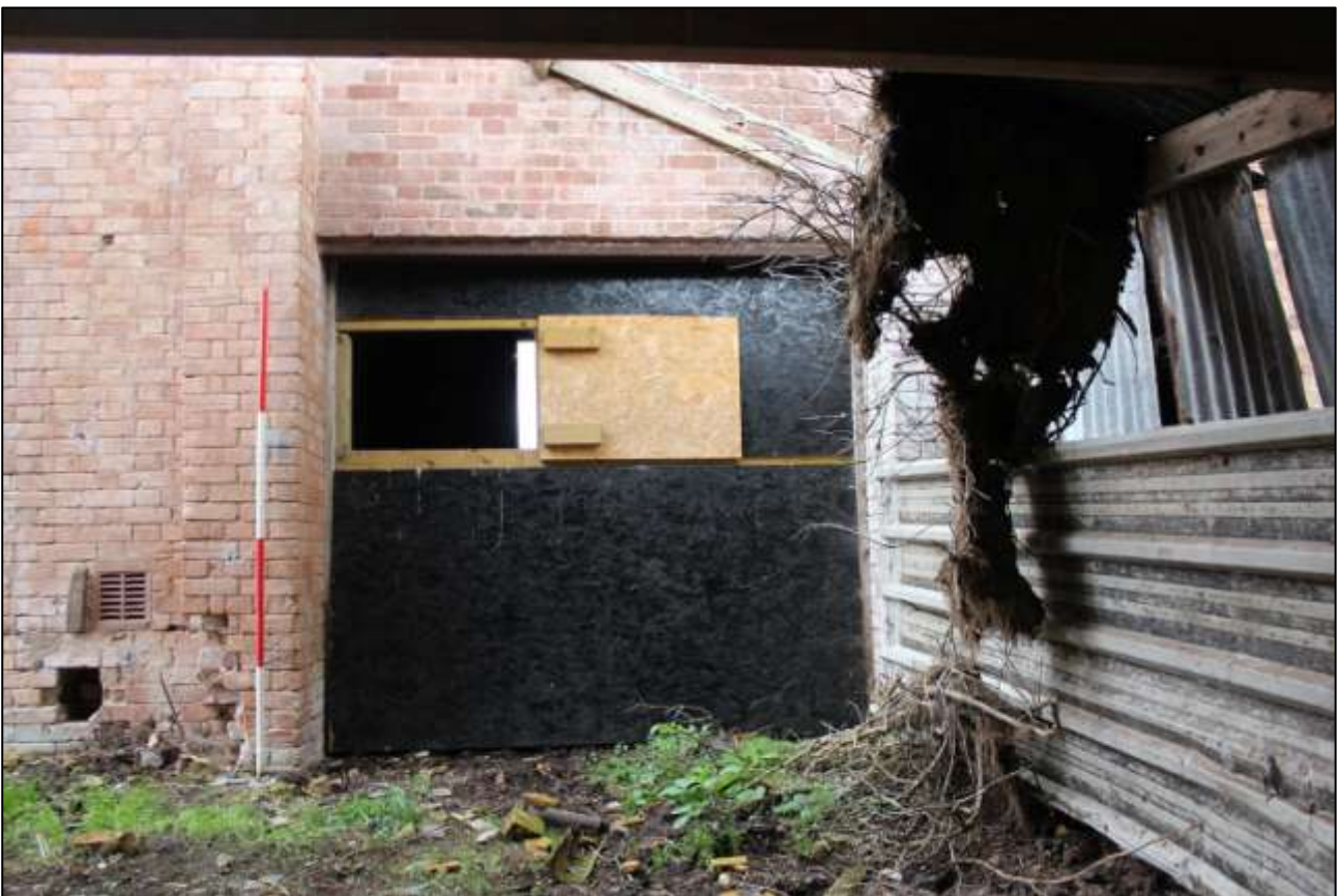
B6 EXTERIOR, WEST WALL, DETAIL OF THE SOUTH WINNOWING DOOR; VIEWED FROM THE WEST (SCALE 2M).
