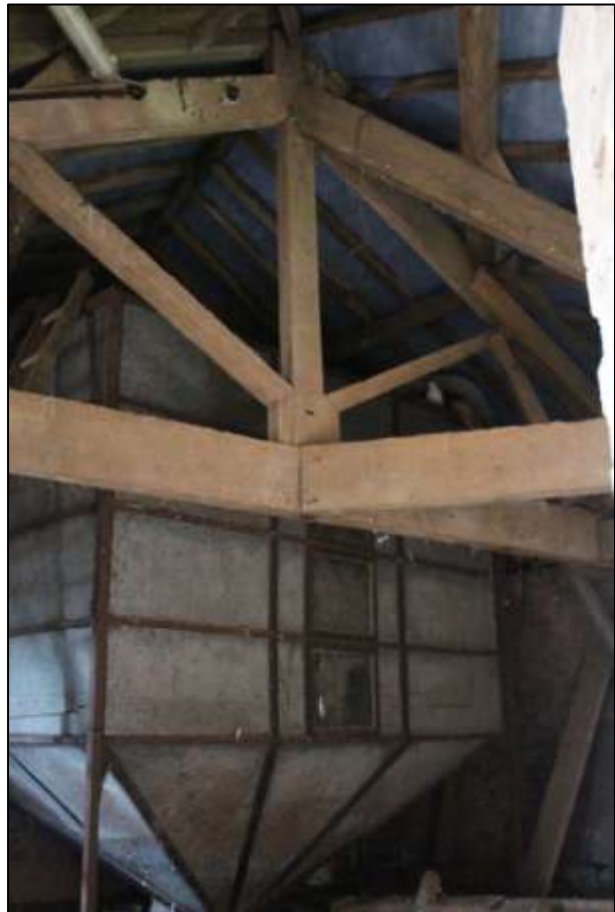
RIGHT: B5 FF INTERIOR, DETAIL OF THE FEED HOPPER AND THE KINGPOST ROOF STRUCTURE; VIEWED FROM THE NORTH-EAST.
