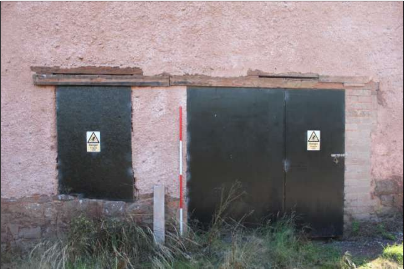
B1 EXTERIOR, NORTH ELEVATION, DETAIL OF D3 AND W4; VIEWED FROM THE NORTH (SCALE 2M).
