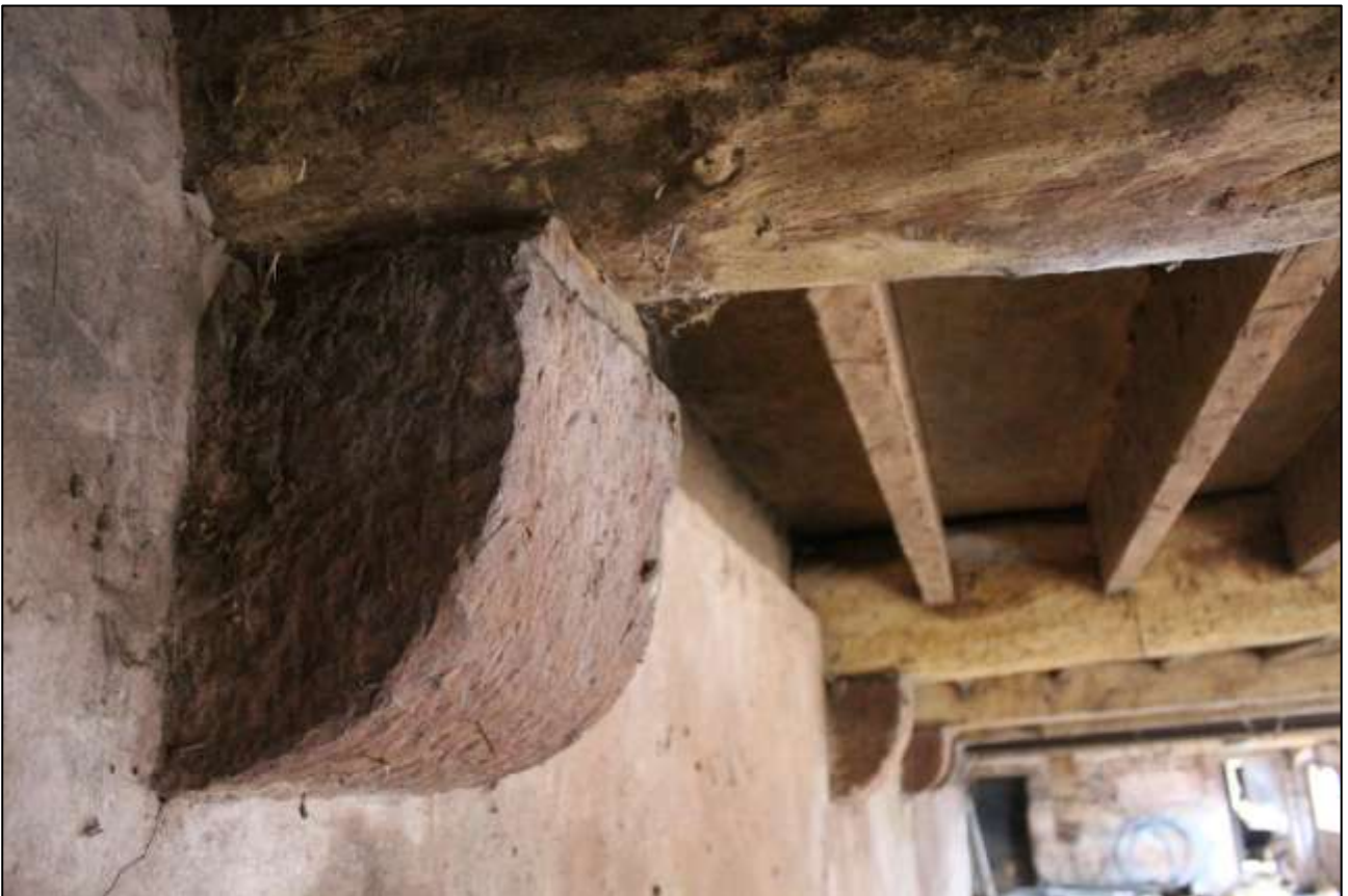
B6 GF INTERIOR, DETAIL OF ONE OF THE CORBELS SUPPORTING THE BEAMS; VIEWED FROM THE SOUTH.
