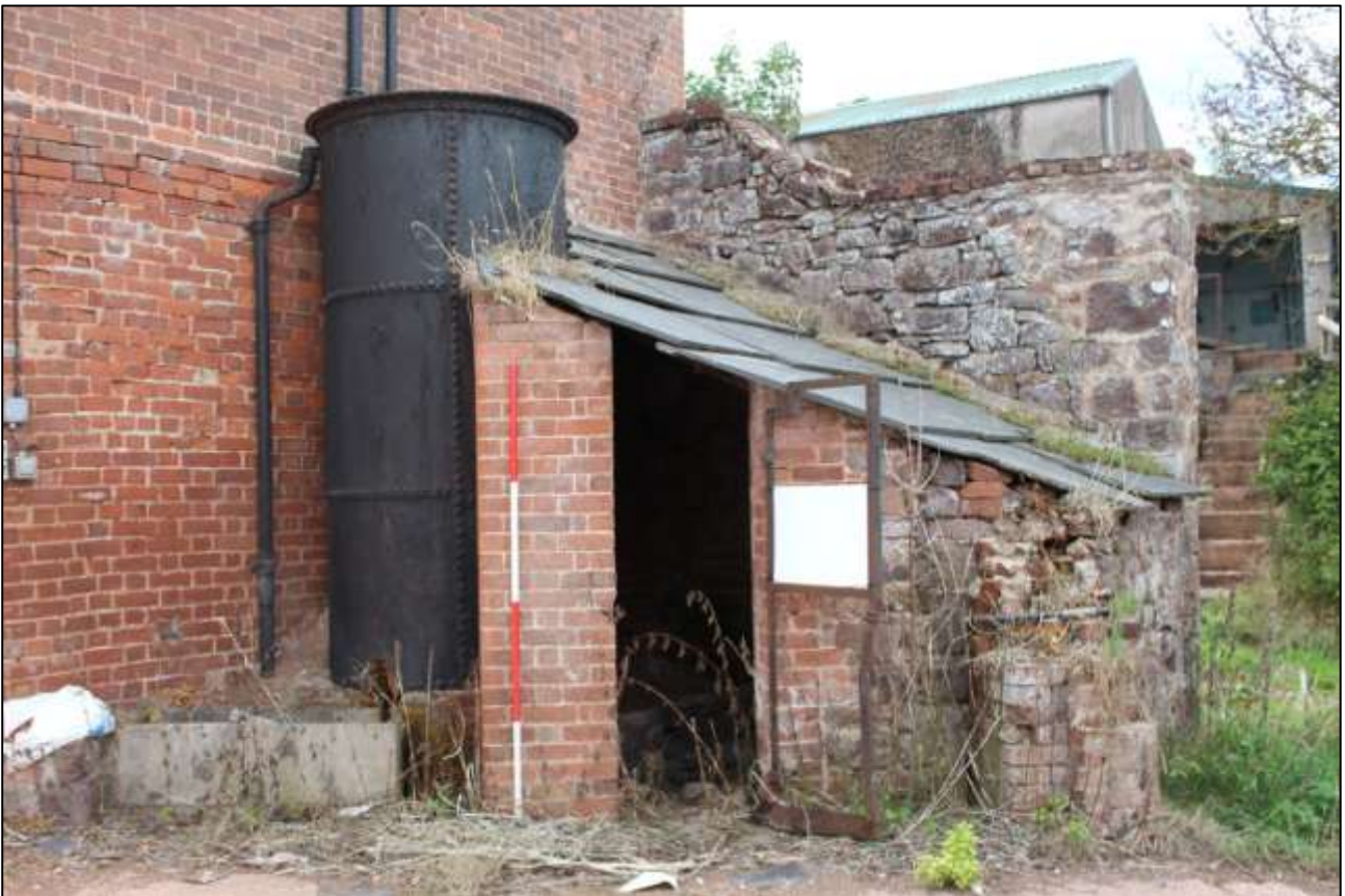
B3, EXTERIOR ELEVATION, EAST WALL AND BOILER; VIEWED FROM THE EAST (SCALE 2M).
