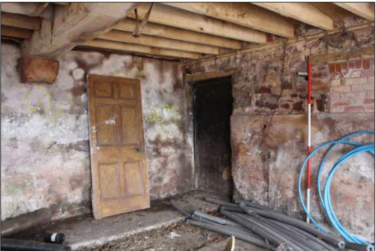
AS ABOVE; VIEWED FROM THE SOUTH-EAST. NOTE THE EX SITU DOMESTIC DOOR FROM THE FARMHOUSE.
