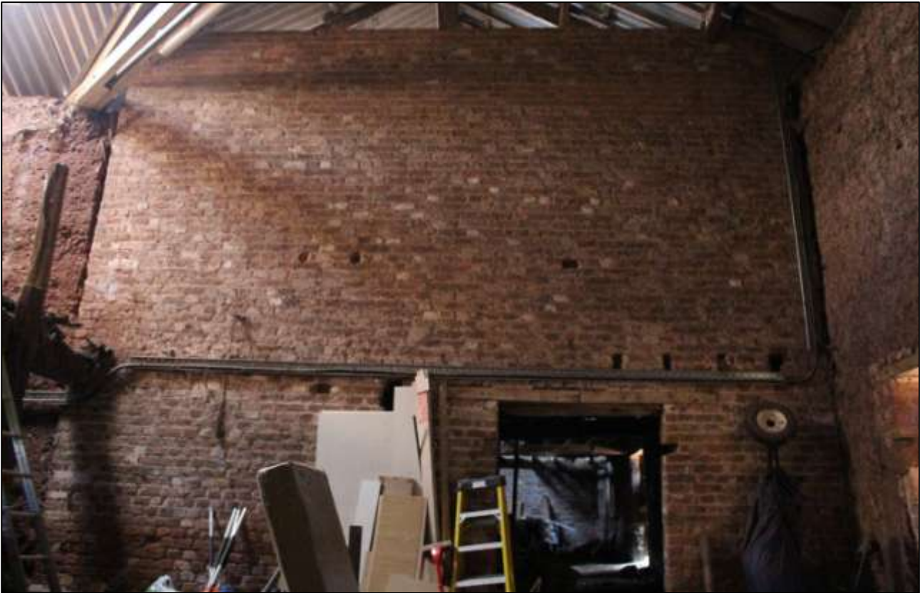
B1 GF INTERIOR, SHOWING THE BRICK WALL BETWEEN B1 AND B2; VIEWED FROM THE NORTH.
