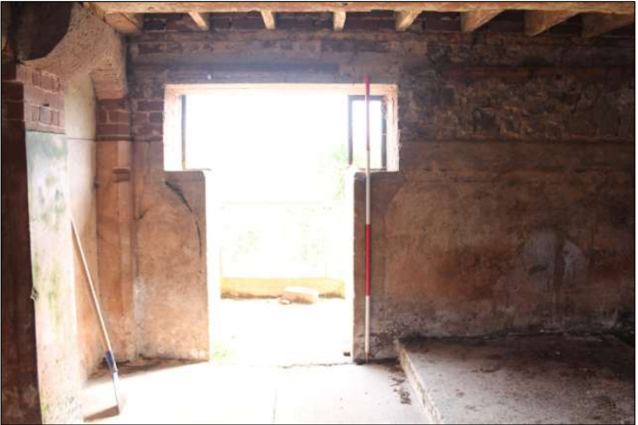
B6 GF INTERIOR, THE FORCED DOORWAY IN THE SOUTH WALL (SCALE 2M); VIEWED FROM THE NORTH.
