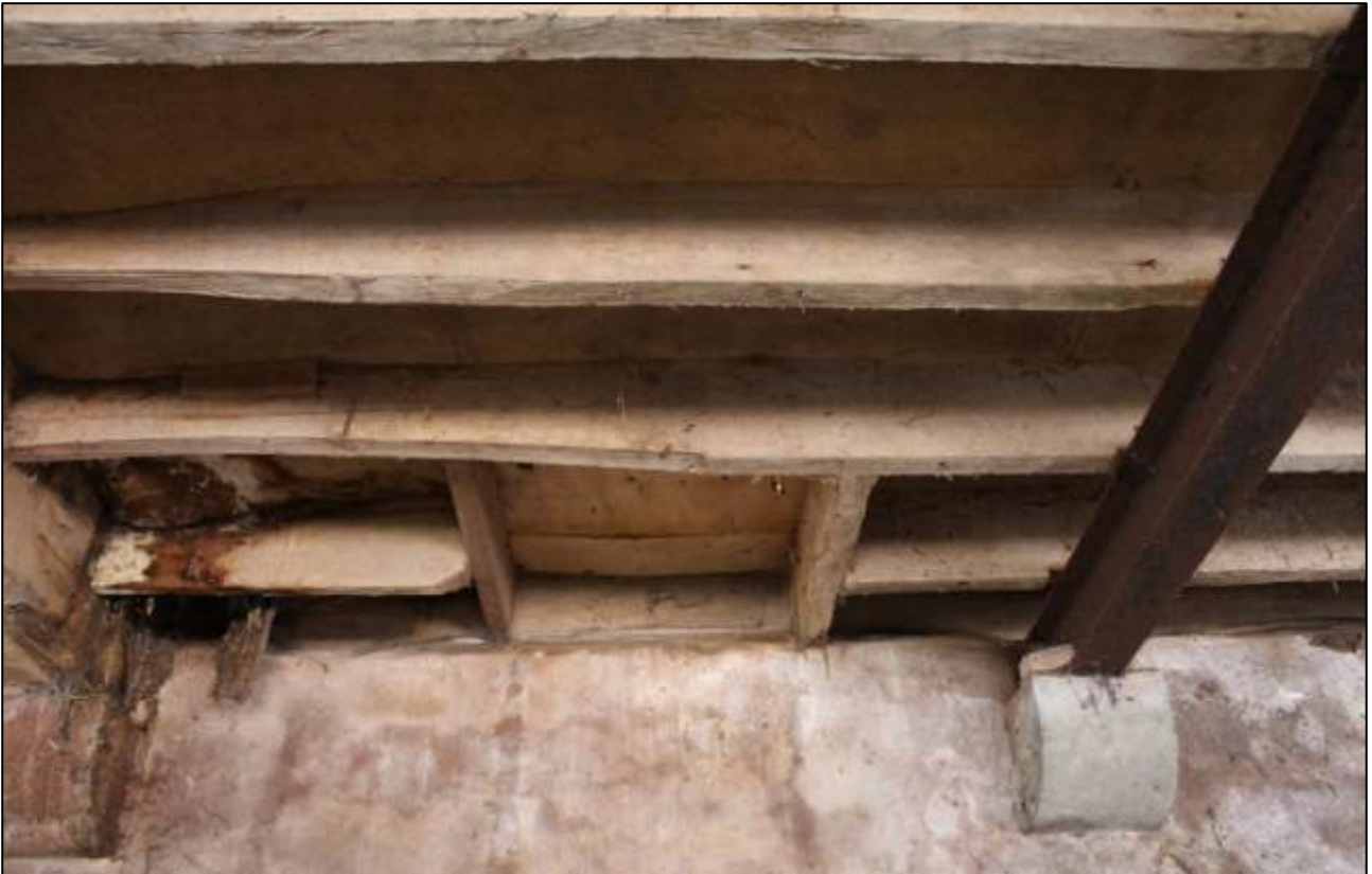
B6 GF INTERIOR, DETAIL OF A HATCH IN THE CEILING; VIEWED FROM THE EAST.
