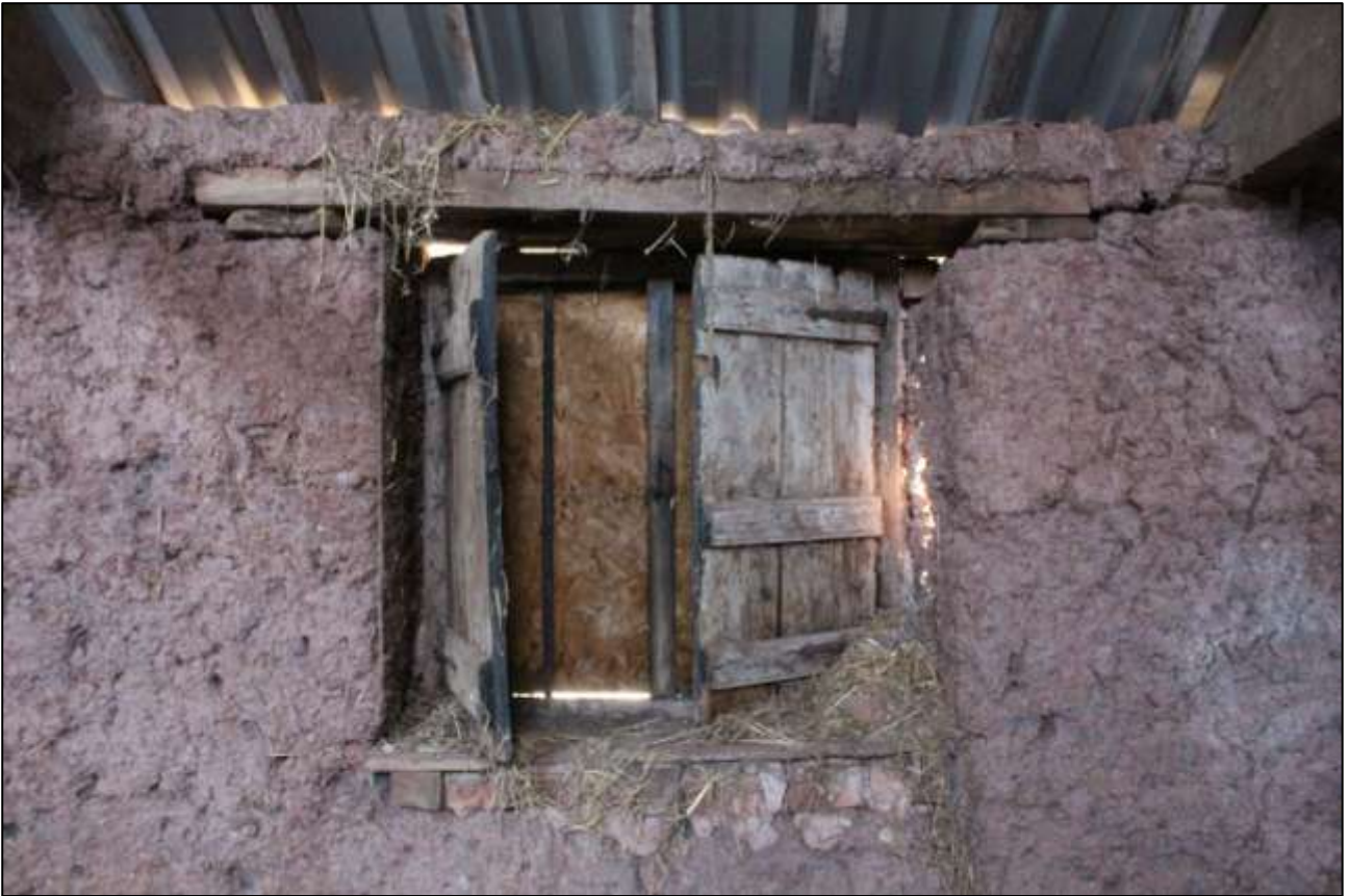
B2 FF INTERIOR, WEST WALL, DETAIL OF W13; VIEWED FROM THE EAST.
