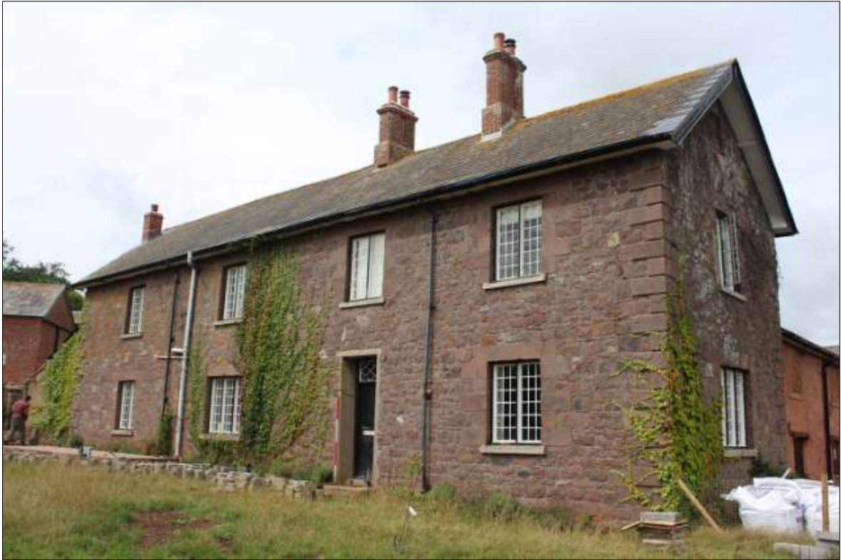
FIGURE 28: THE SOUTH ELEVATION OF THE FARMHOUSE; VIEWED FROM THE SOUTH-EAST (SCALE 2M).
