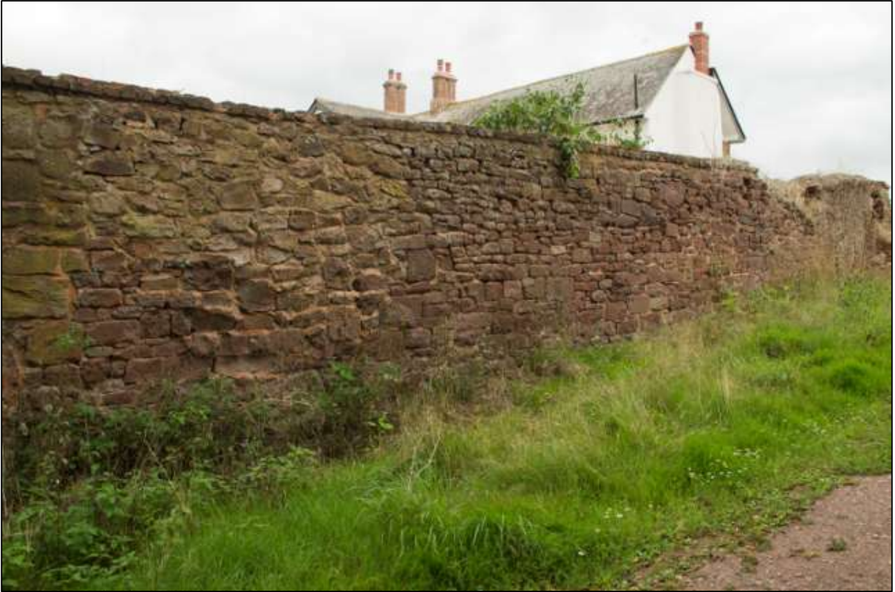
THE WALL OF THE YARD ATTACHED TO THE REAR OF THE FARMHOUSE, NOTE THE GOOD QUALITY STONEWORK; VIEWED FROM NORTH-WEST.
