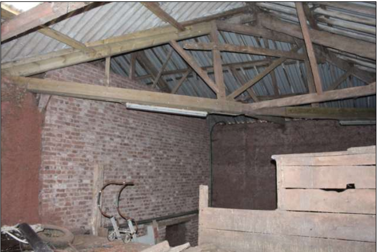
B1 FF INTERIOR, SHOWING THE BRICK WALL BETWEEN B1 AND B2; VIEWED FROM THE NORTH-EAST.
