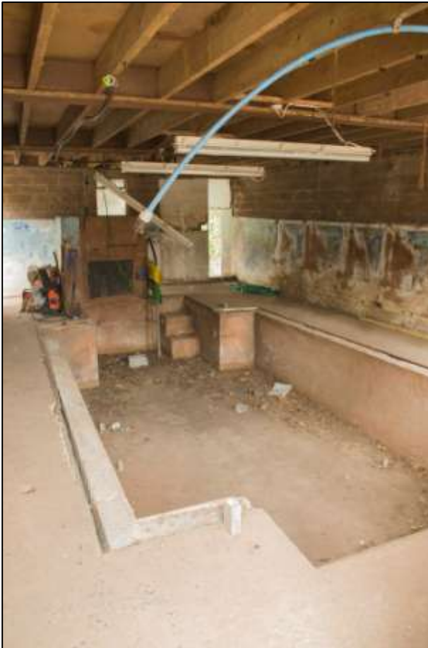
B12, THE INTERIOR OF THE MODERN MILKING PARLOUR; VIEWED FROM THE SOUTH-WEST.
