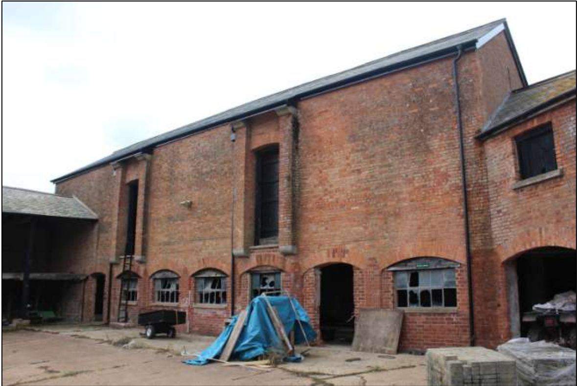
FIGURE 21: THE EAST ELEVATION OF THE B6 THE THRESHING BARN; VIEWED FROM THE NORTH-EAST (SCALE 2M).
