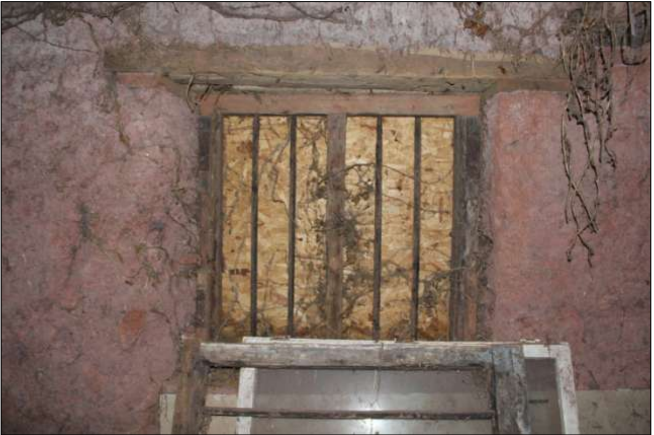
B2 GF INTERIOR, EAST WALL, DETAIL OF W10; VIEWED FROM THE WEST.
