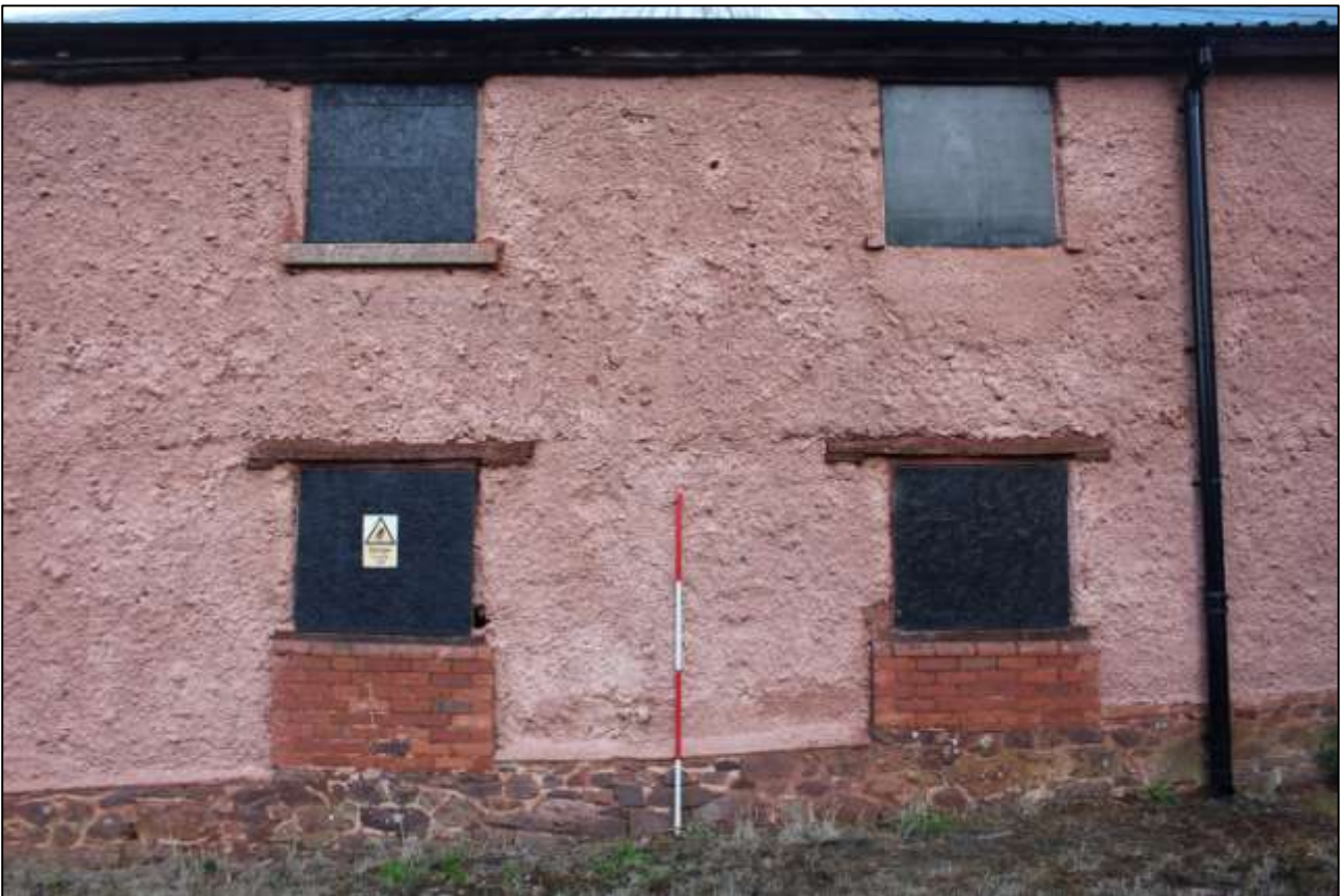
B2 EXTERIOR, WEST ELEVATION, SHOWING W2, W3, W12 AND W13; VIEWED FROM THE WEST (SCALE 2M).
