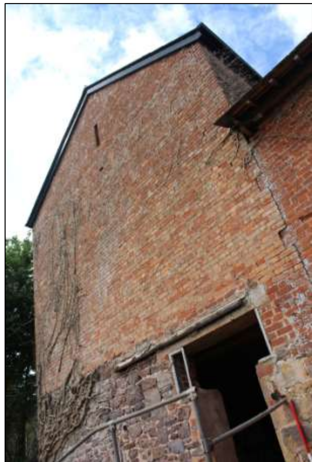
RIGHT: B6 EXTERIOR, SOUTH WALL, SHOWING THE TALL BLIND ELEVATION; VIEWED FROM THE SOUTH-EAST (SCALE 2M).
