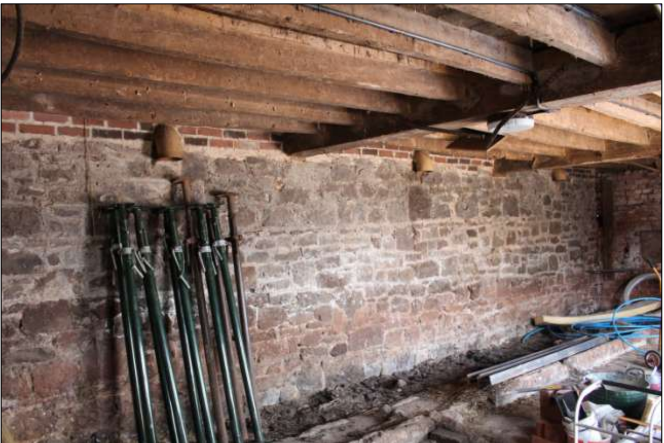
B4A INTERIOR, SHOWING THE ROUGHLY-COURSED EXTERIOR STONE YARD WALL; VIEWED FROM THE SOUTH.
