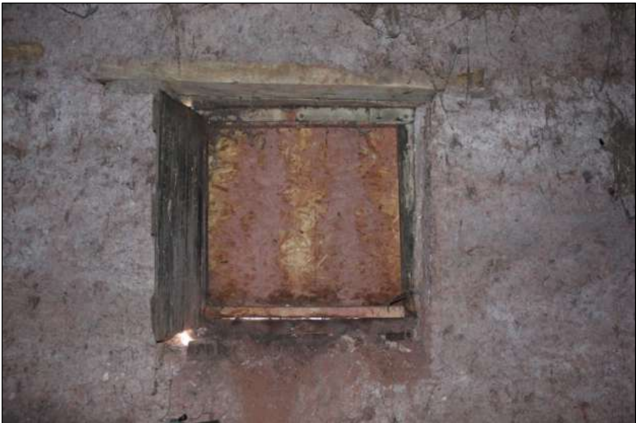
B2 GF INTERIOR, WEST WALL, DETAIL OF W3; VIEWED FROM THE EAST.
