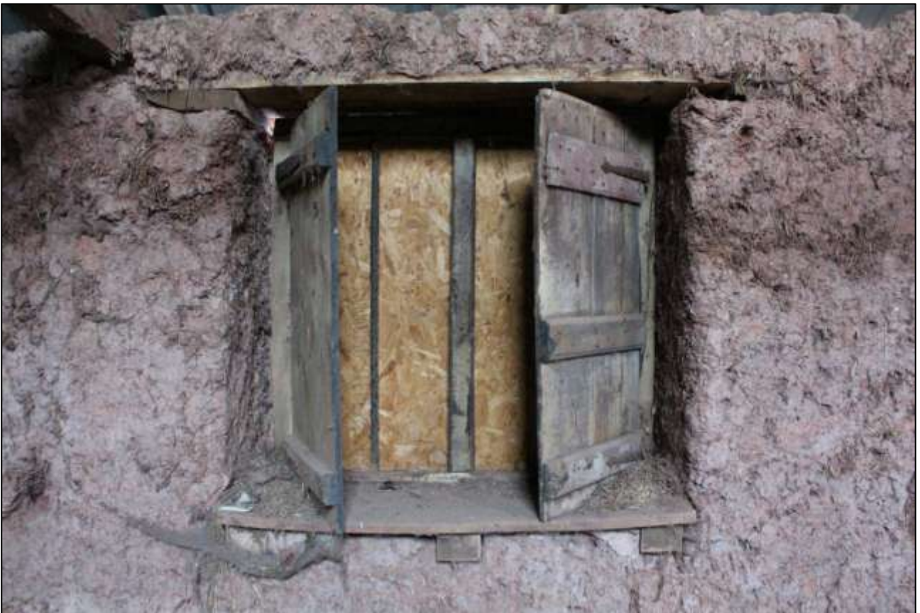
B2 FF INTERIOR, WEST WALL, DETAIL OF W11 ; VIEWED FROM THE EAST.
