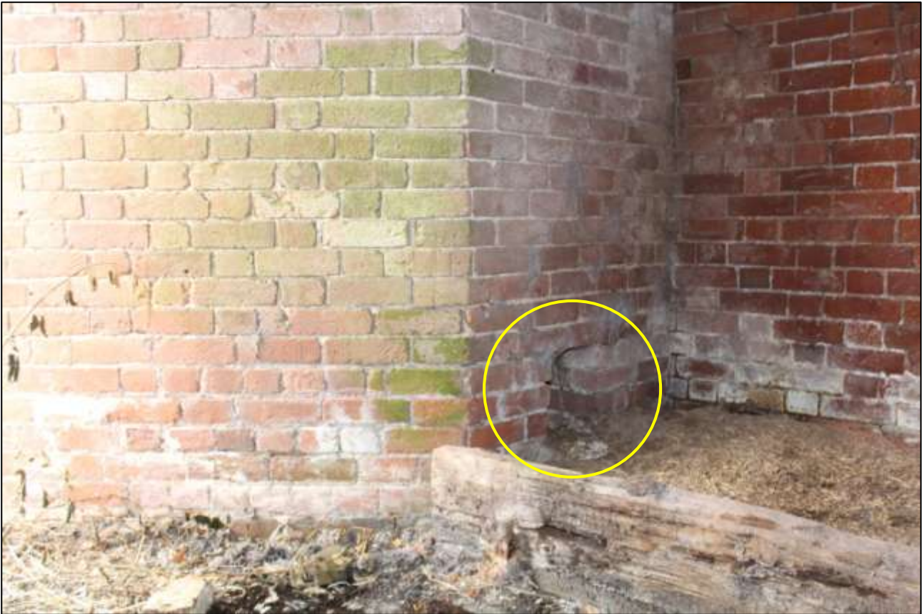
AS ABOVE, WITH FLASH ILLUMINATING THE STOKE HOLE (INDICATED).
