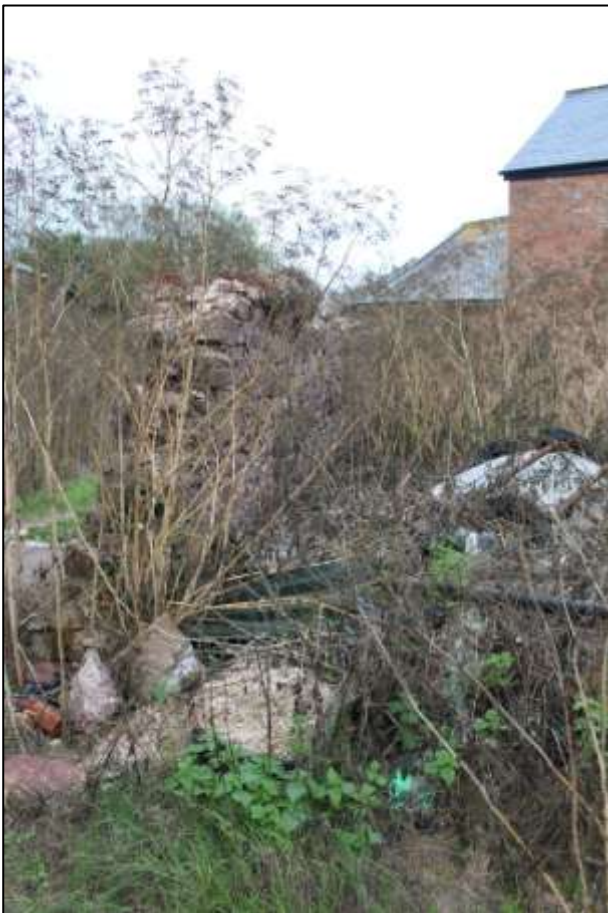
B9 EXTERIOR, VIEW OF THE UTILISED STONE YARD WALL; VIEWED FROM THE SOUTH-WEST.
