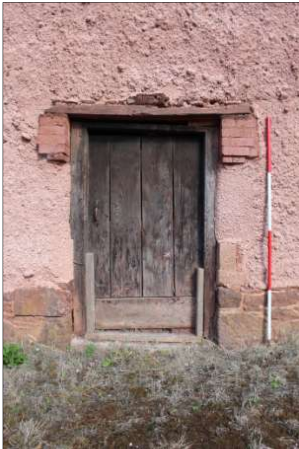
LEFT: B1 EXTERIOR, DETAIL OF D2; VIEWED FROM THE WEST (SCALE 2M).
