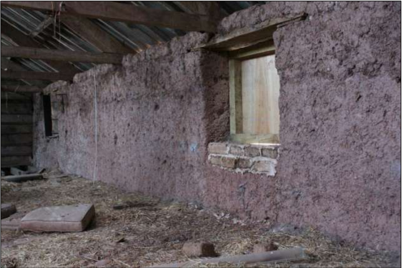
B2 FF INTERIOR, WEST WALL, SHOWING W12 AND W11 AND RAISES IN THE COB; VIEWED FROM THE NNE.
