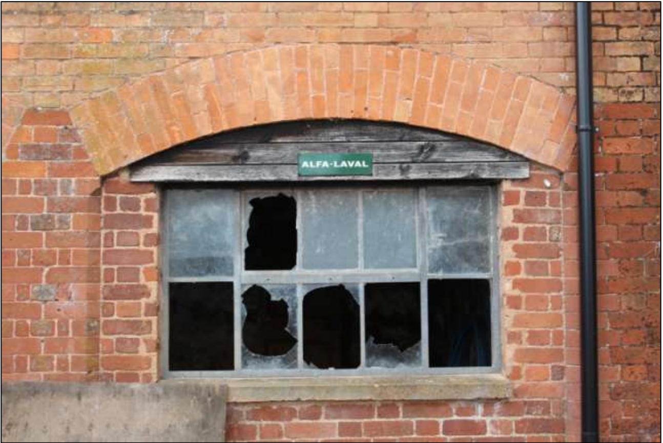
B6 EXTERIOR, EAST WALL, DETAIL OF THE CRITTAL-STYLE WINDOW AND ALFA LAVAL SIGN; VIEWED FROM THE EAST.
