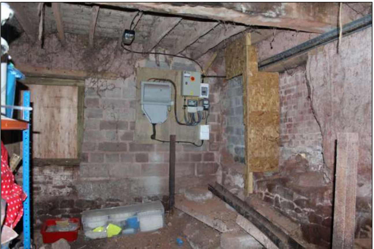
B1 GF INTERIOR, EAST WALL SHOWING W6 AND W7; VIEWED FROM THE WEST.
