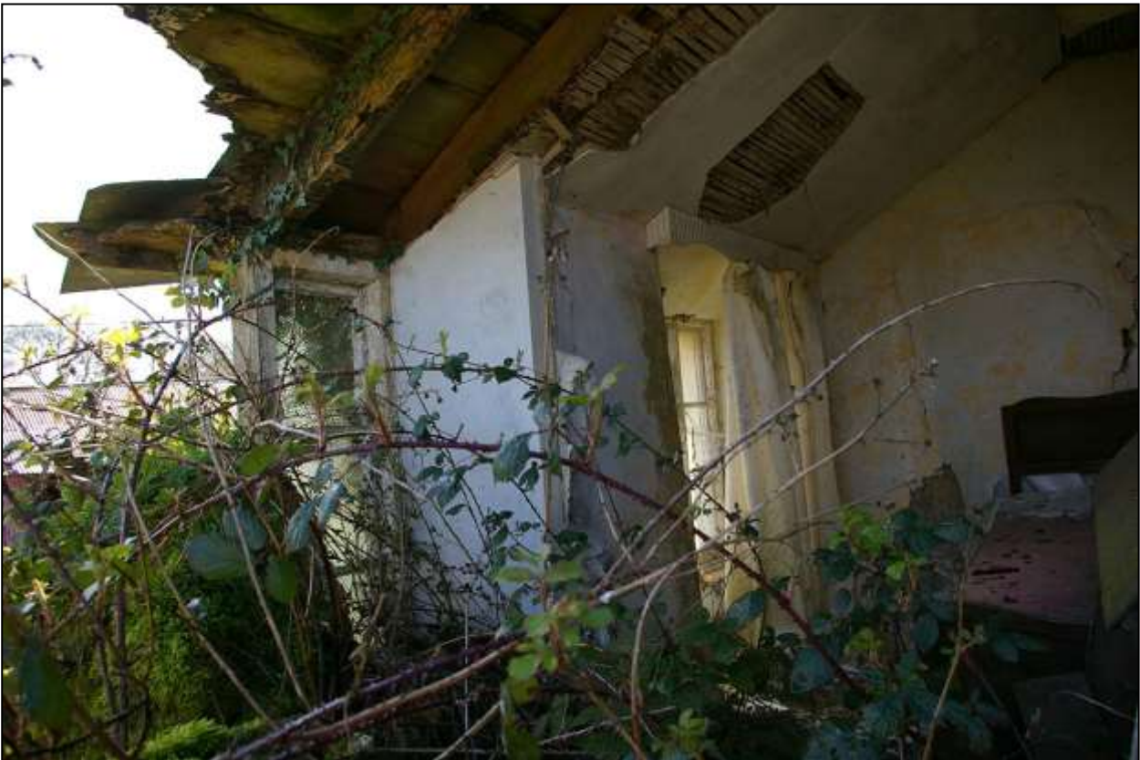
116. VIEW INTO R11 FROM THE NORTH-EAST, SHOWING THE TWO WINDOWS; THE LATE 19 TH /EARLY 20 TH CENTURY ROOF AND CEILING CONSTRUCTION ARE VISIBLE. VIEWED FROM THE NNE.
