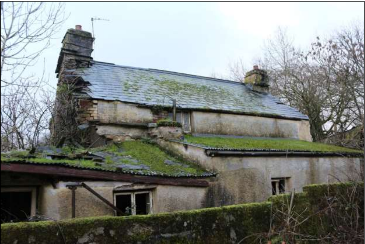
14. REAR ELEVATION OF FARMHOUSE WITH LEAN-TOS; R5 IS IN HIGHER PART TO RIGHT, R6 IS IN LOWER PART TO LEFT; VIEWED FROM THE NNE.
