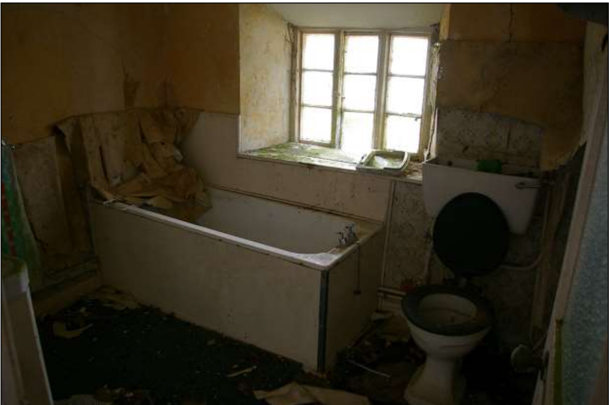
122. R10, WITH 19 TH CENTURY THREE-LIGHT CASEMENT (W13) AND MID-20 TH CENTURY BATHROOM FITMENTS. VIEWED FROM THE EAST.
