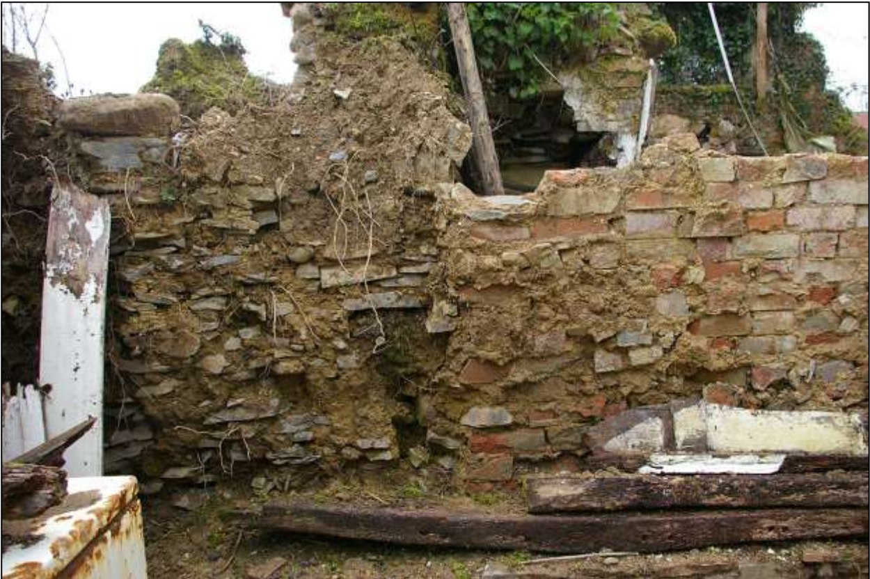
110. R7, THE REAR SIDE OF STONE AND BRICK RE-FACING OF THE (NOW LOST) COB WALL; THE LOOSE TIMBERS IN THE FOREGROUND ARE RESTING ON THE STONE RUBBLE PLINTH OF THE COB WALL. VIEWED FROM THE NORTH-WEST.
