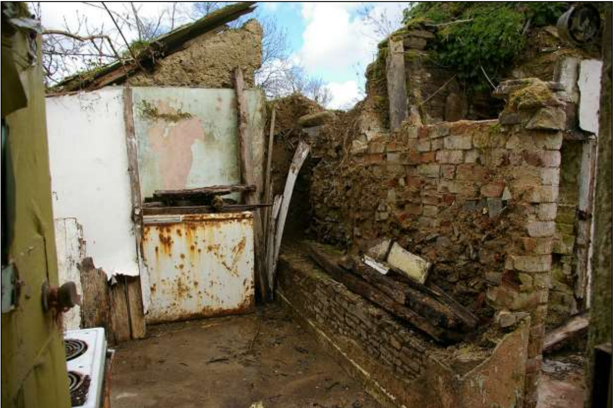
108. R7 FROM THE DOOR TO R6, SHOWING THE MEDIEVAL STONE AND COB REAR WALL OF R2, PARTLY REPLACED BY BRICK TO ITS SOUTH-EASTERN FACE. THICK COB WALL FORMS THE NORTH-EAST END OF R8. VIEWED FROM THE WSW.
