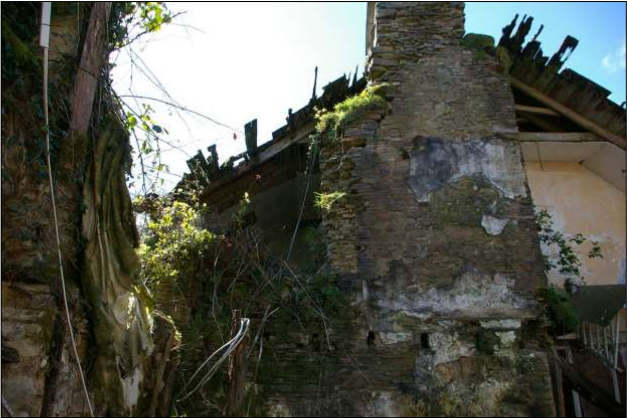
115. ROOM VOIDS FLANKING AXIAL STACK, LOOKING FROM R2. R11 TO THE LEFT, R9 TO THE RIGHT. VIEWED FROM THE NORTH-EAST.
