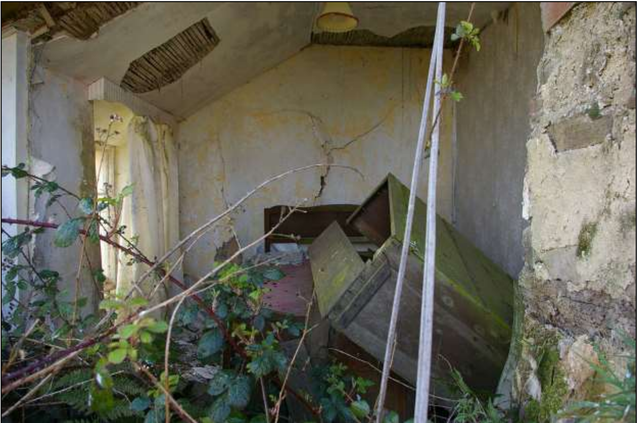
117. R11 FROM R2, DIRECTLY ABOVE R3 WHERE THE CEILING HAS COLLAPSED. TIMBER LACING AND PLASTER IN THE SIDE OF THE CHIMNEY STACK TO THE RIGHT (POSSIBLE CUPBOARD?). VIEWED FROM THE NORTH-EAST.
