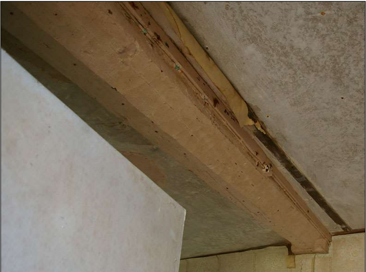
82. THE DEEP-CHAMFERED NORTHERN SIDE OF THE NORTHERN BEAM IN R3. NOTE THE ADZE MARKS. VIEWED FROM THE ENE.
