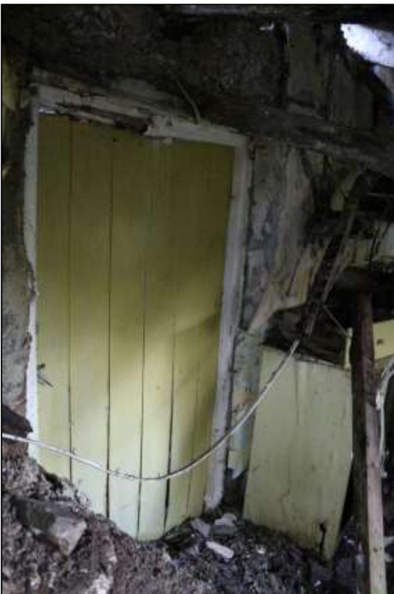
31. LEFT: REAR DOOR TO CROSS PASSAGE FROM R6 (D3); VIEWED FROM THE NORTH.
