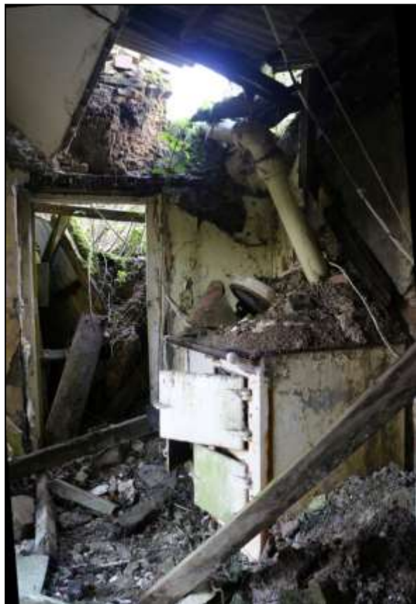
32. RIGHT: COLLAPSED EAST END OF R6 WITH 20 TH CENTURY AGA; VIEWED FROM THE SOUTH-WEST.
