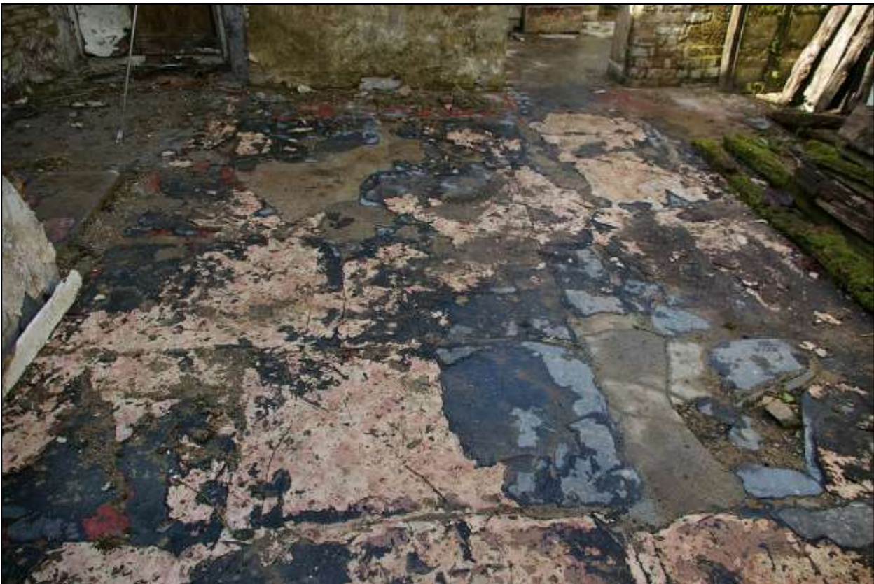
72. VIEW OF THE HEAVY SLATE SLAB FLAGSTONE FLOOR, OF VERY FINE QUALITY BUT MUCH DAMAGED AND PATCHED, WITHIN R2; VIEWED FROM THE SOUTH-EAST.
