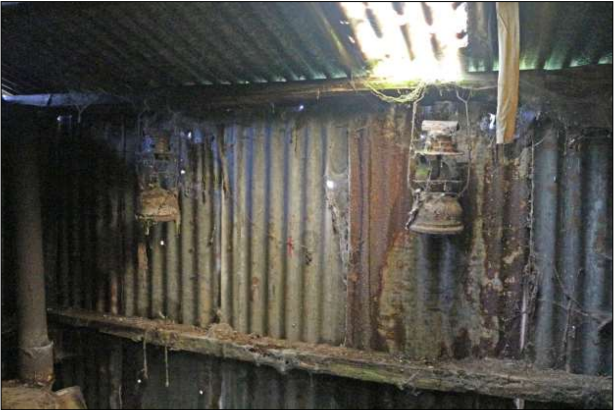
45. TILLEY LAMPS HANGING ON THE NORTH-EAST WALL OF THE CORRUGATED IRON LEAN-TO; VIEWED FROM THE SOUTH.
