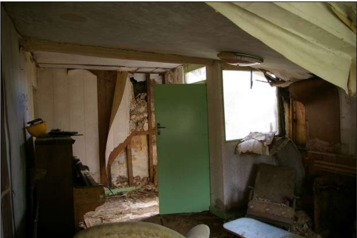
78. R3, SHOWING THE BOARDED NORTH WALL WITH BLOCKED DOORWAY TO R5, PARTITION AND DOOR (D6) TO STAIR LOBBY R2B AND MOULDED NORTHERN BEAM. VIEWED FROM THE SOUTH.
