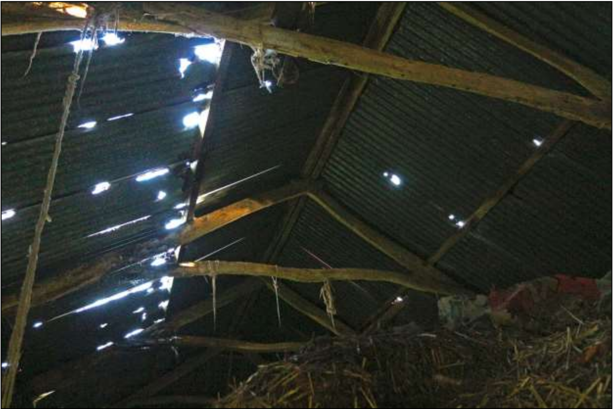
130. ROOF STRUCTURE OF LINHAY. ROUGHLY DRESSED ROUNDWOOD TRUSSES FORMERLY SUPPORTING SLATES. SAWN PURLINS & CORRUGATED IRON ARE MID-20 TH CENTURY. VIEWED FROM THE WEST.
