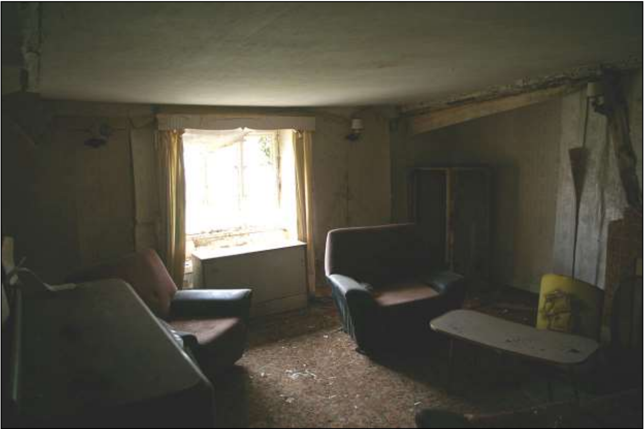
86. R4, SHOWING WINDOW TO SOUTH FRONT AND TRANSVERSE BEAMS TO UPPER LEFT AND RIGHT; VIEWED FROM THE SOUTH.
