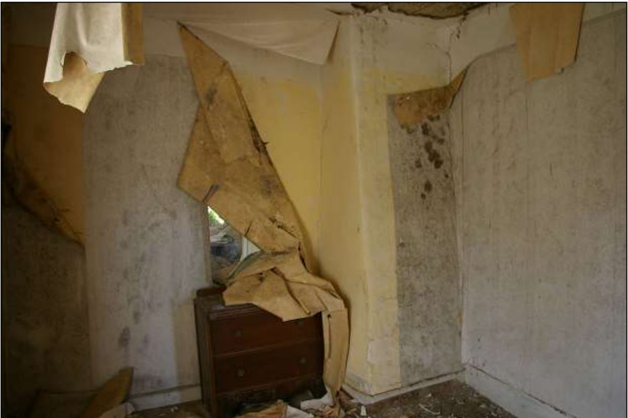
124. SOUTH-WEST WALL OF R12 WITH TAPERED CHIMNEY BREAST; VIEWED FROM THE EAST.
