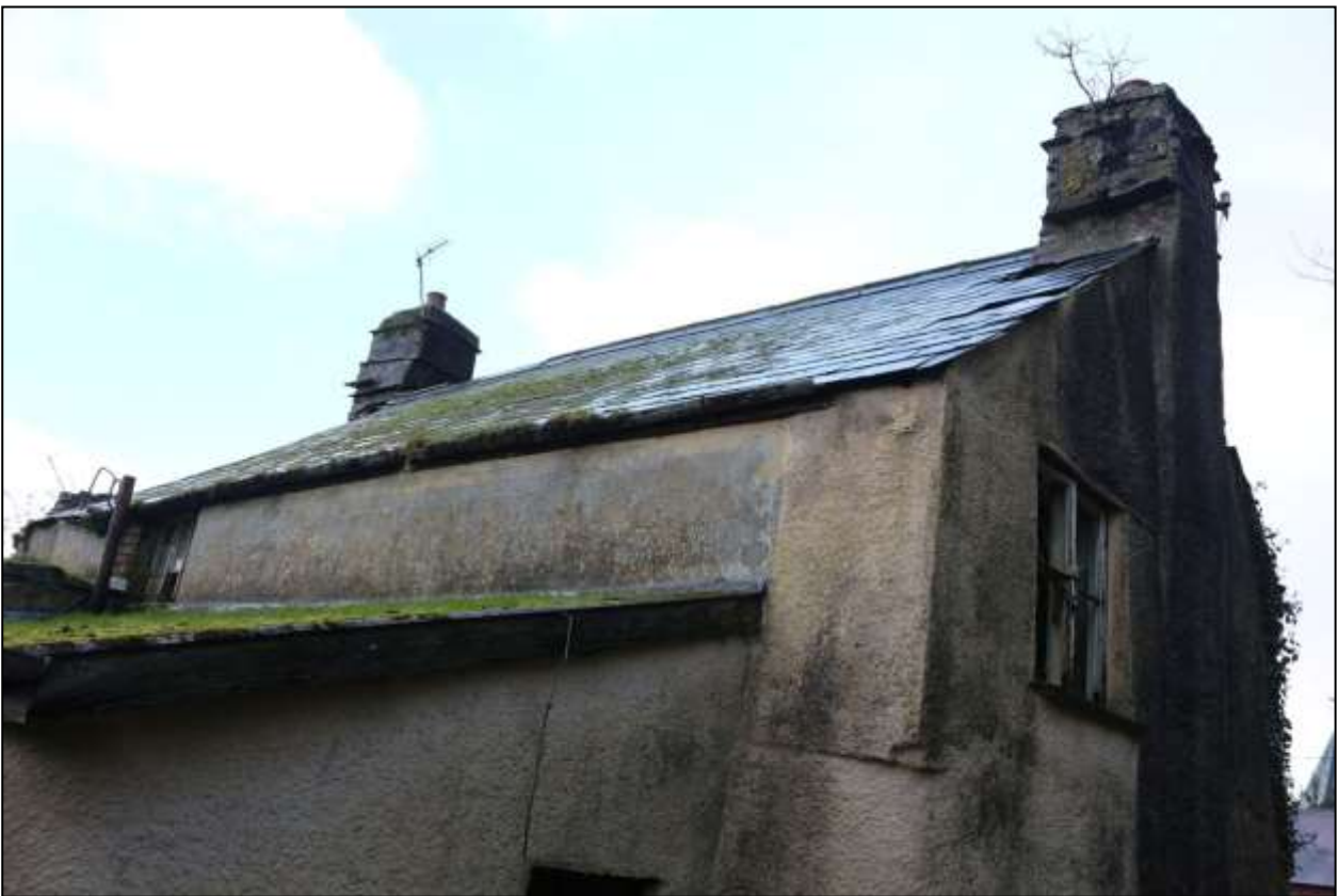
18. NORTH-WEST CORNER OF HOUSE. CURVED CORNER FORMERLY CONTAINED NEWEL STAIRCASE OF 17 TH CENTURY DATE. REGULAR CORNER ABOVE IS PROBABLY A BRICK REPAIR. WINDOW (W12) LIGHTS FIRST FLOOR R13. NOTE RAISED WEATHERING ON CHIMNEY AT TOP RIGHT FOR FORMER THATCH ROOF COVERING. VIEWED FROM THE NORTH-WEST.
