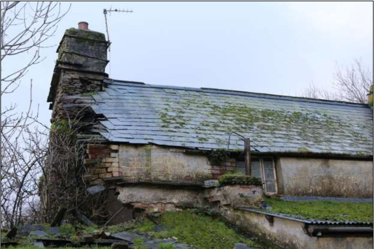
15. LATE 19 TH OR EARLY 20 TH CENTURY BRICKWORK ON REAR WALL OF STAIRCASE 2B, REPLACING THIN FAILED COB WALLING. NOTE SMALL BLOCKED WINDOW (BO5), PREVIOUSLY LIGHTING STAIRCASE AND UPPER LANDING. VIEWED FROM THE NORTH.
