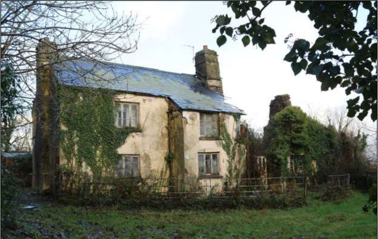
1. SOUTH-EAST ELEVATION BEFORE CLEARANCE; VIEWED FROM THE SOUTH. NOTE RAILINGS ENCLOSING FRONT GARDEN.
