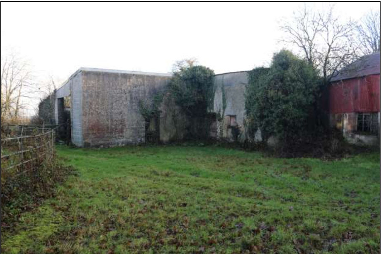
131. L-PLAN BUILDINGS AT EASTERN CORNER OF FARMYARD. FORMER COTTAGE WITH COB CONSTRUCTION TO CENTRE. VIEWED FROM THE WEST.
