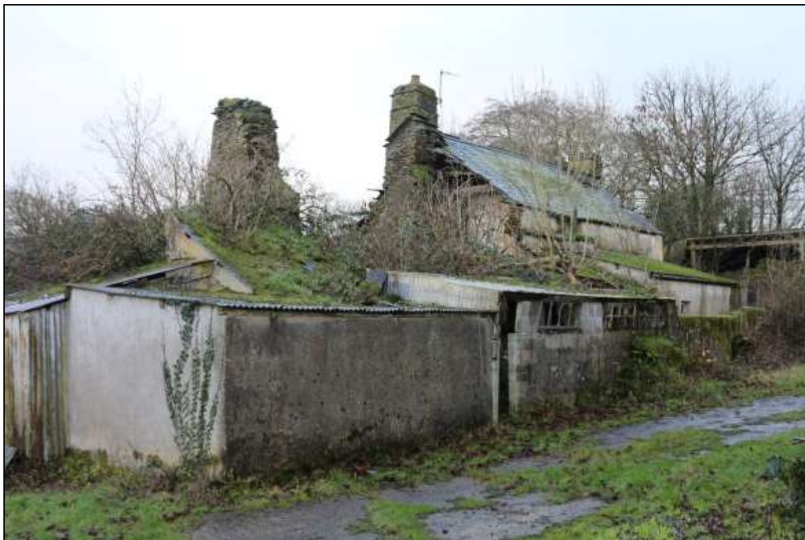
FIGURE 8: THE REAR ELEVATION OF THE FARMHOUSE AT TOWN BARTON SHOWING THE LEAN-TO ADDITIONS; FROM THE NORTH.
