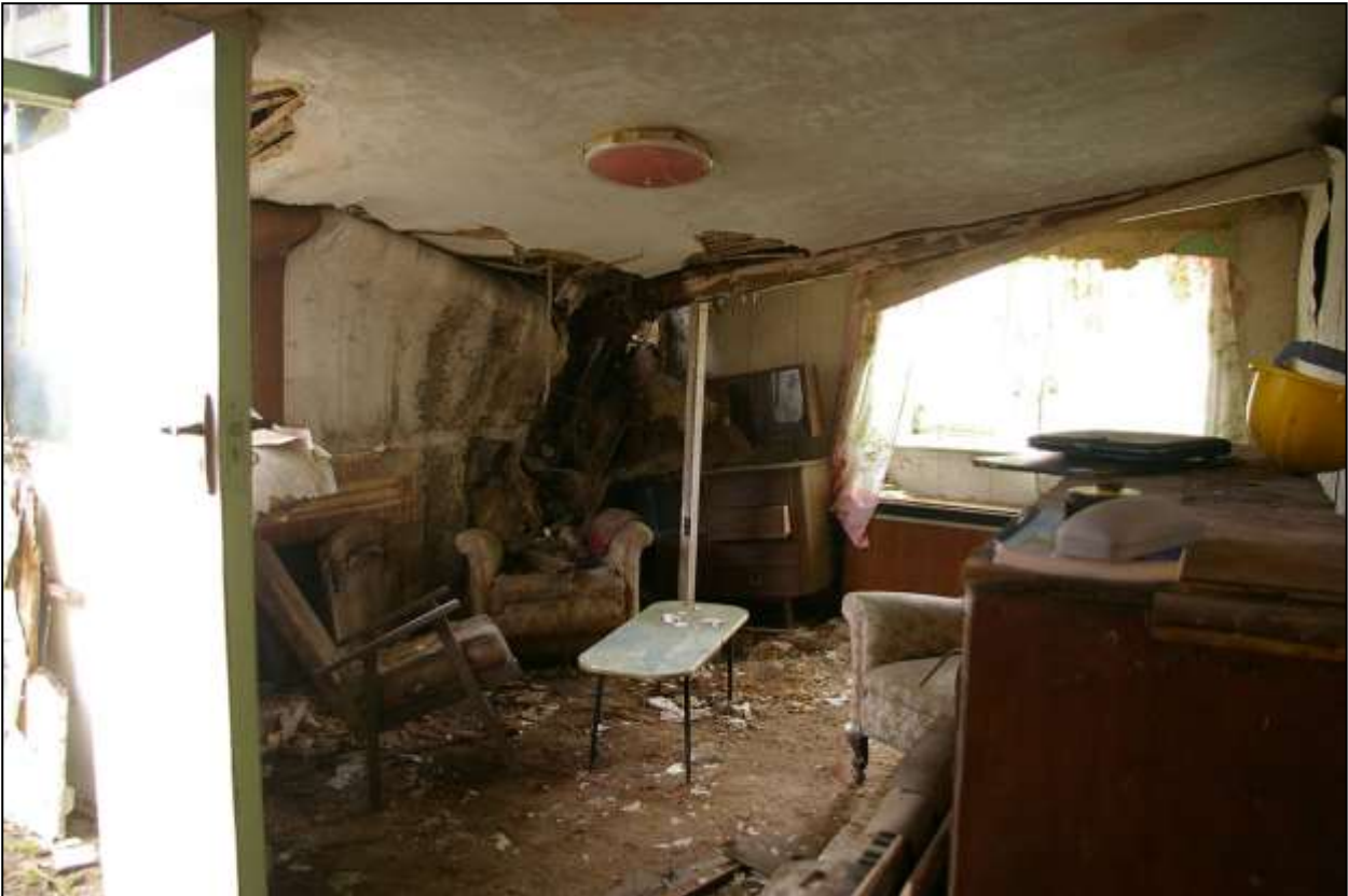
73. R3, SHOWING THE CEILING COLLAPSE IN THE SOUTH-EAST CORNER; VIEWED FROM THE WSW.
