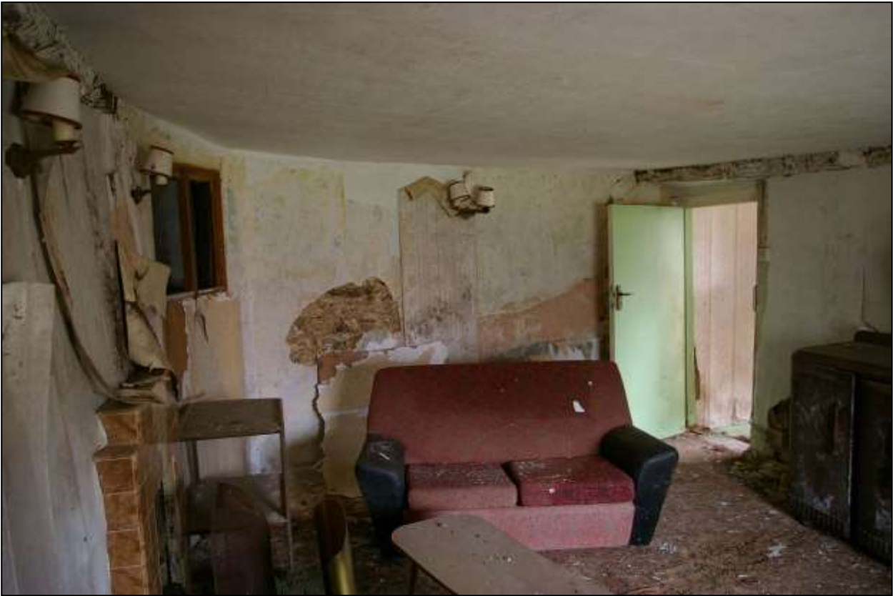
92. R4, WITH CUPBOARD ON SITE OF WINDER STAIR ON LEFT AND DOOR TO R3 ON RIGHT. NOTE MASONRY IN NORTH WALL WHERE PLASTER HAS FALLEN OFF ABOVE SOFA. VIEWED FROM THE SOUTH-EAST.
