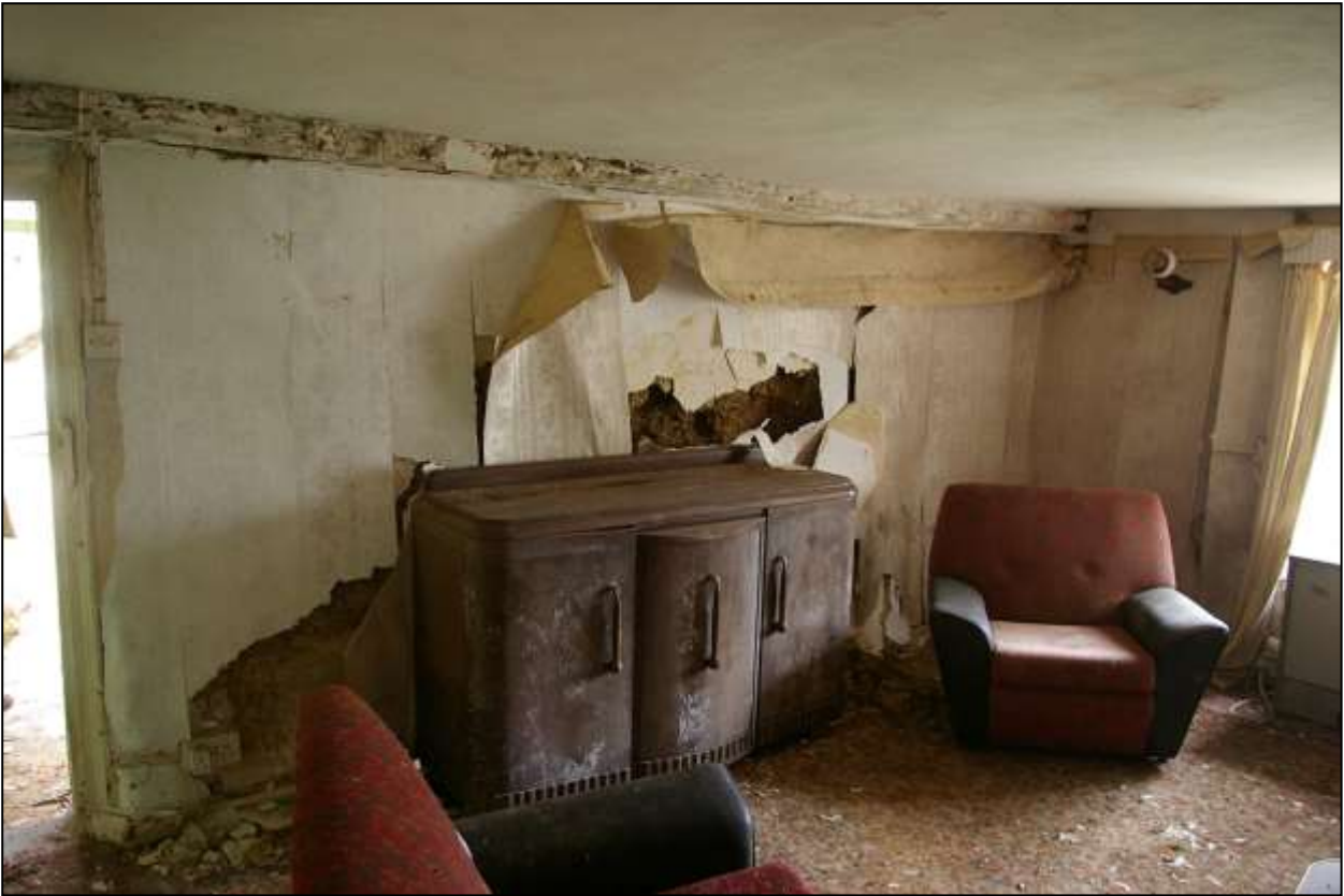
90. NORTH-EAST WALL OF R4. NOTE COB EXPOSED WHERE PLASTER HAS FALLEN AWAY. VIEWED FROM THE NORTH-WEST.
