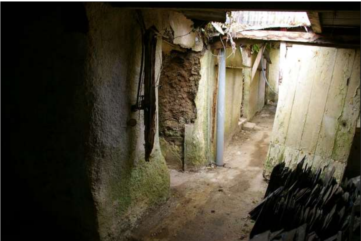
111. LOOKING SOUTH-WEST ALONG THE THICK COB OUTER WALL OF THE OUTSHUTS CONTAINING R7 AND R8. THIS WAS AN OUTSIDE WALL UNTIL CONCRETE FARM BUILDINGS WERE BUILT AGAINST IT IN THE 1950S. VIEWED FROM THE NORTH-EAST.
