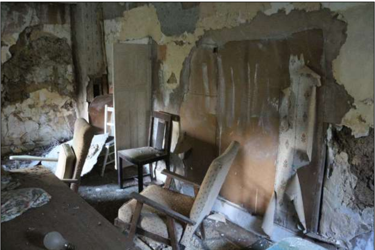
25. DETAIL OF REAR WALL OF HOUSE ON SOUTH SIDE OF R5. LARGE BLOCKED OPENING BEHIND HARDBOARD IN FOREGROUND, 18 TH CENTURY PANELLED SHUTTERS RECYCLED AS DOOR TO CUPBOARD BEYOND. BOXING IN CORNER FOR 20 TH CENTURY FLUE PIPE. VIEWED FROM THE WEST.
