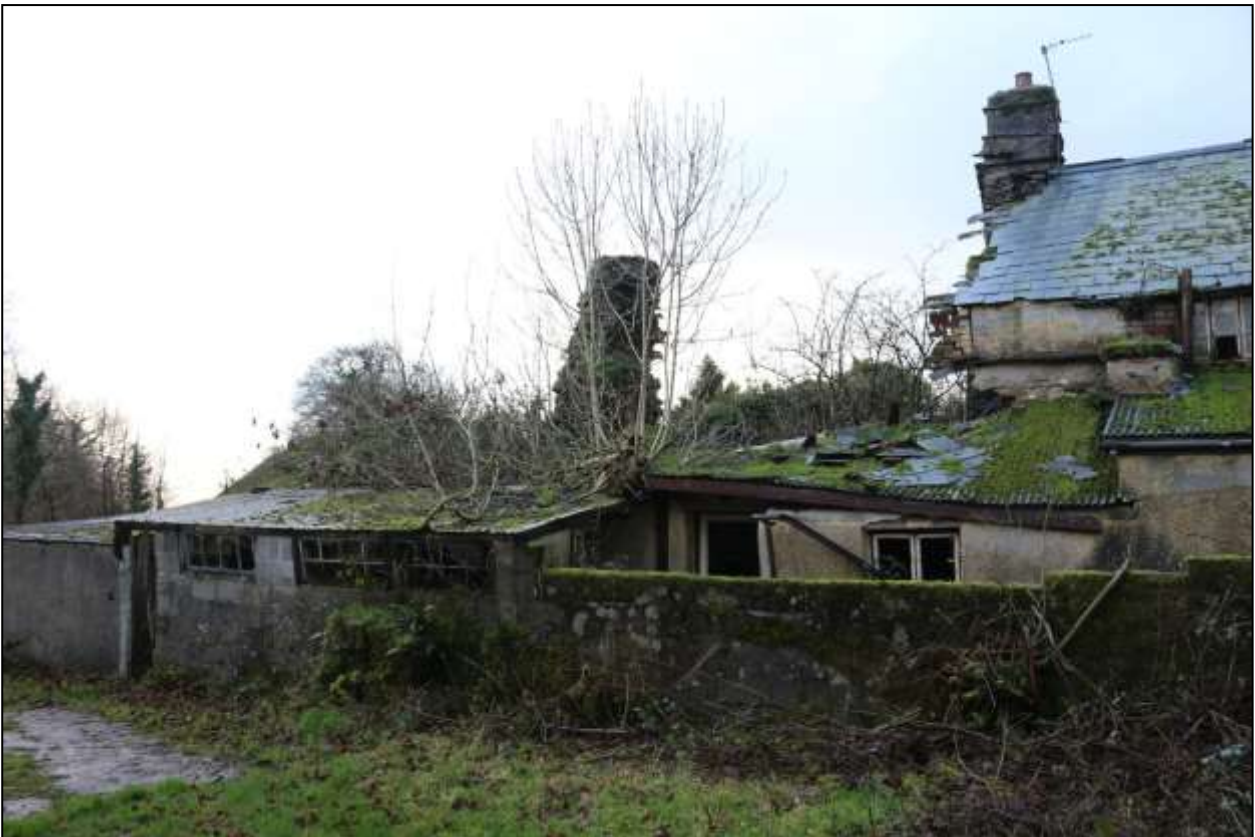
16. GENERAL VIEW OF COLLAPSED EASTERN HALF OF HOUSE. SEMI-COLLAPSED LEAN-TO IN RIGHT FOREGROUND CONTAINS R6; R7 LIES IN THE VEGETATION TO LEFT OF ASH TREE GROWING IN ROOF. VIEWED FROM THE NORTH-WEST.
