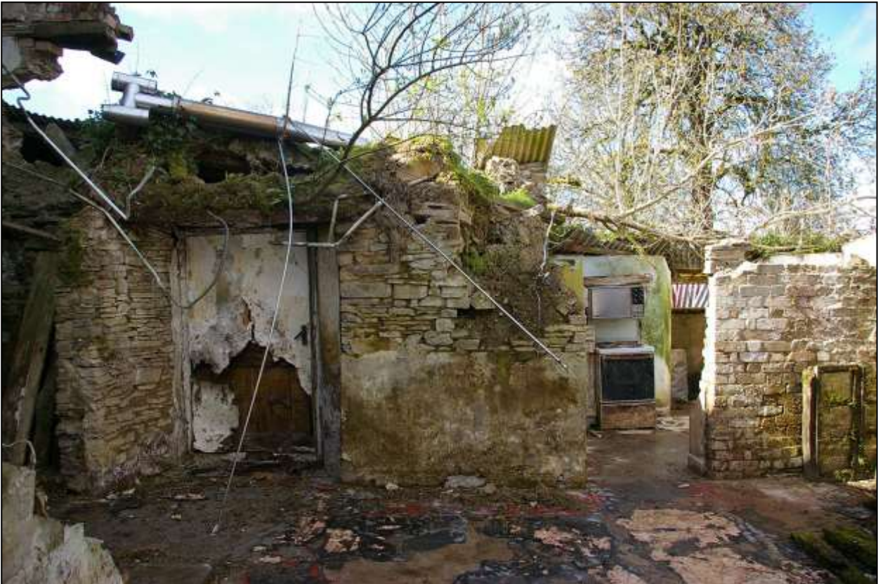
61. REAR (NORTH-WEST) WALL OF R2, SHOWING THE FORMER CROSS PASSAGE DOORWAY ON THE LEFT (D3) AND A LATER DOOR TO R7 ON THE RIGHT (D4). BRICKWORK FACES DECAYED COB. VIEWED FROM THE SOUTH-EAST.
