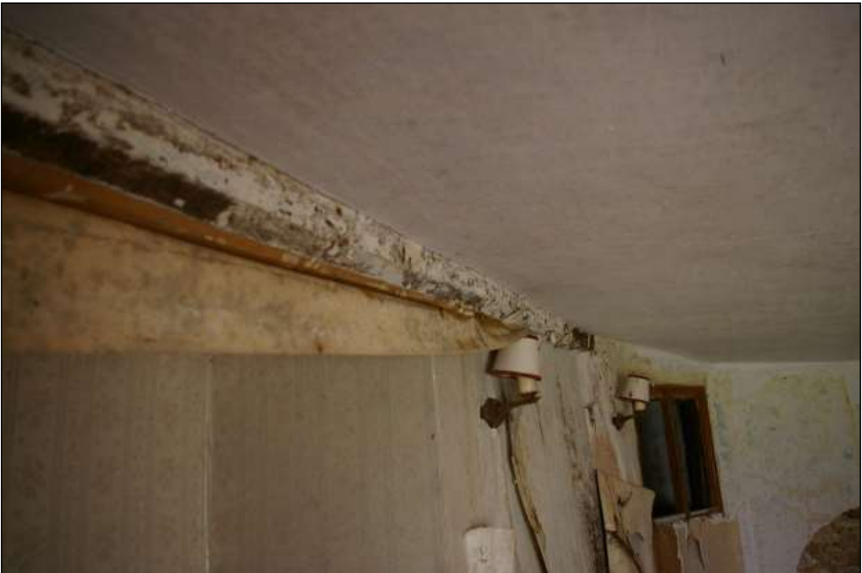
91. DETAIL OF THE NARROW-CHAMFERED CEILING BEAM AGAINST THE CHIMNEY BREAST IN R4; VIEWED FROM THE SOUTH-EAST.
