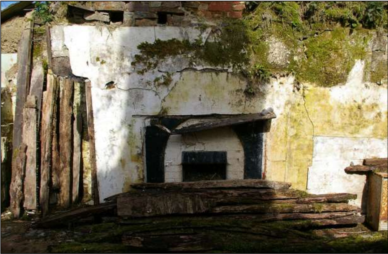
71. VIEW OF THE VICTORIAN FIREPLACE (FP2) SET INTO A MUCH LARGER BLOCKED HEARTH WITH HEAVY CHAMFERED LINTEL, IN THE EASTERN AXIAL STACK THAT SERVES R2. VIEWED FROM THE SOUTH-WEST
