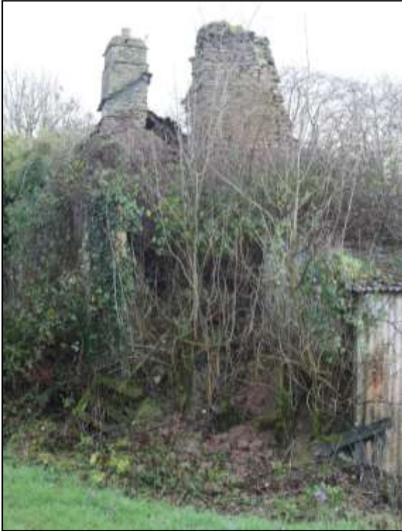
9. WESTWARD VIEW INTO PARTLY COLLAPSED AND OVERGROWN REMAINS OF R1; CREAM-PAINTED FRONT WALL IS JUST VISIBLE IN IVY ON LEFT; VIEWED FROM THE EAST.
