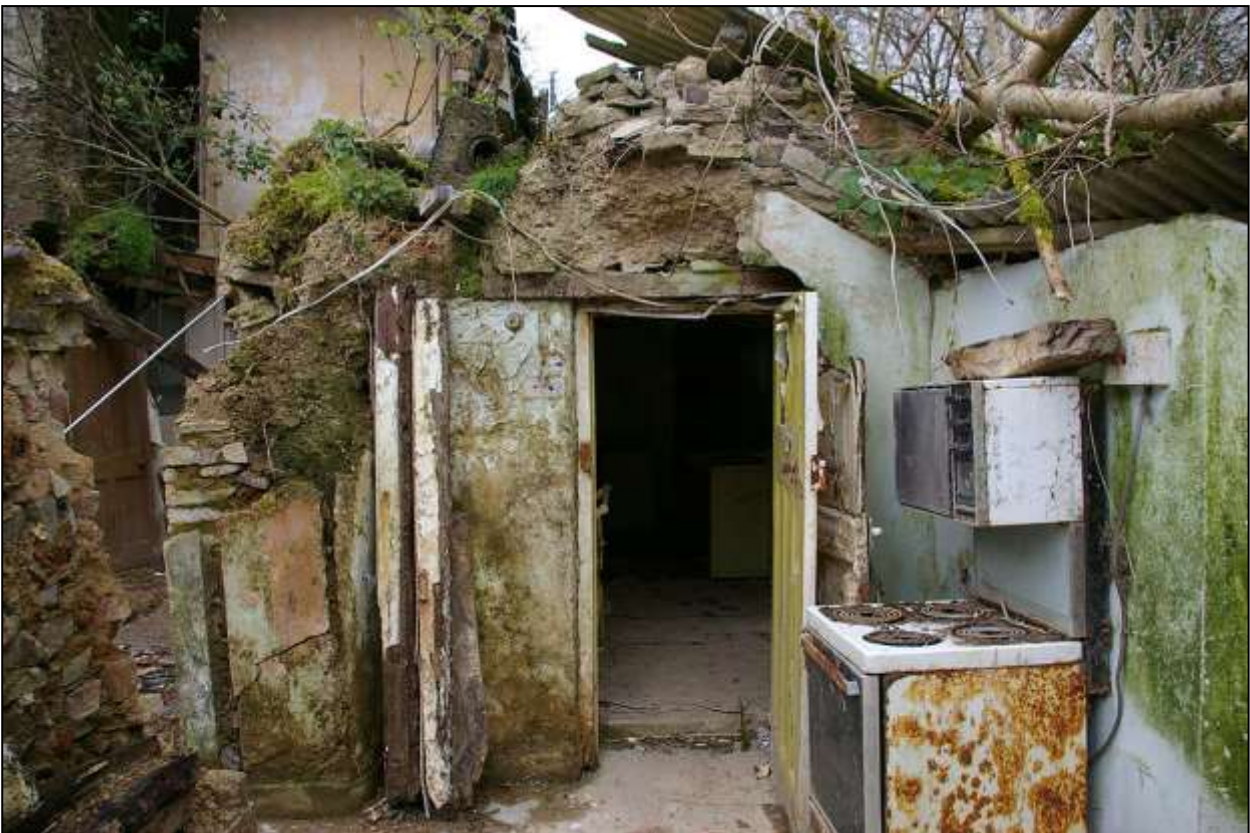
109. R7, WITH LARGELY COLLAPSED MEDIEVAL COB BACK WALL OF HOUSE TO LEFT AND COB DIVIDING WALL ABOVE DOOR TO R6 IN CENTRE (D11). VIEWED FROM THE NORTH-EAST.
