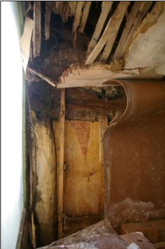
75. DETAIL OF WEST SIDE OF FIREPLACE IN R3, SHOWING HEAVY CHAMFERED TIMBER LINTEL AND GRANITE UPRIGHT SUPPORT; VIEWED FROM THE SOUTH-WEST.
