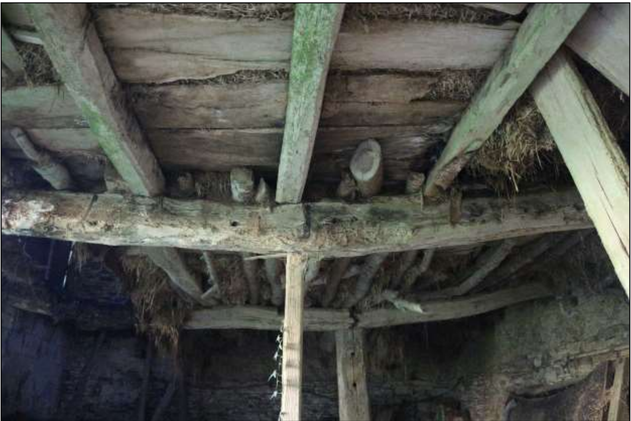
129. GROUND FLOOR OF LINHAY. NOTE RUBBLE WALLS SUPPORTING COB UPPERS. TRANSVERSE BEAMS PRIMARY, PERHAPS CHAMFERED JOISTS ALSO, BUT ROUNDWOOD IS LATER. CONCRETE WALL TO LEFT INFILLS FORMERLY OPEN FRONTAGE. VIEWED FROM THE WEST.
