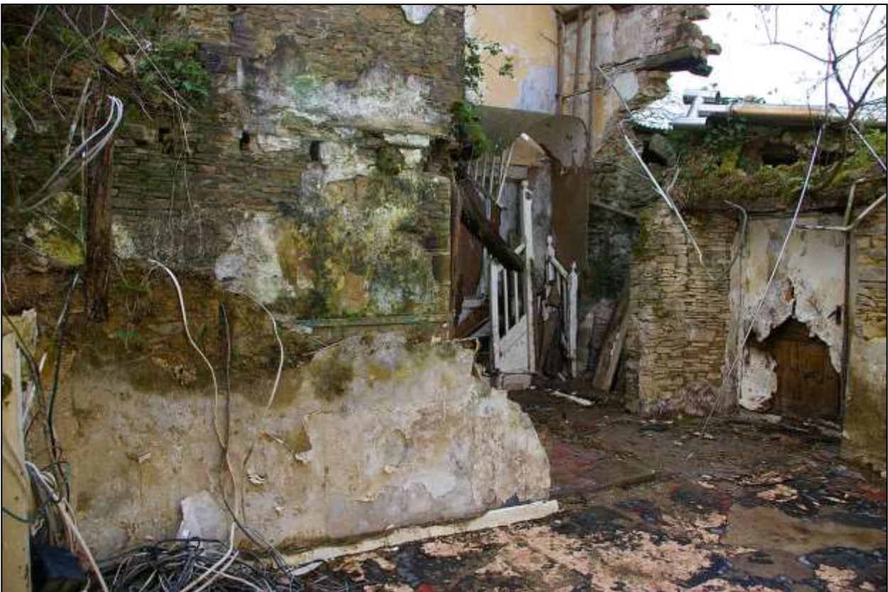
62. VIEW OF THE RUBBLE AXIAL CHIMNEY STACK FORMING THE NORTH-WEST WALL OF THE CROSS PASSAGE R2b. PART OF ITS EASTERN PARTITION TO R2 CAN BE SEEN IN THE LEFT FOREGROUND. NOTE MASONRY PIER PROJECTING BEYOND LINTEL TO LEFT OF CROSS-PASSAGE REAR DOOR. LOBBY BEYOND CONTAINS REMAINS OF LATE 17 TH -EARLY 18 TH CENTURY STAIRCASE. VIEWED FROM THE EAST.
