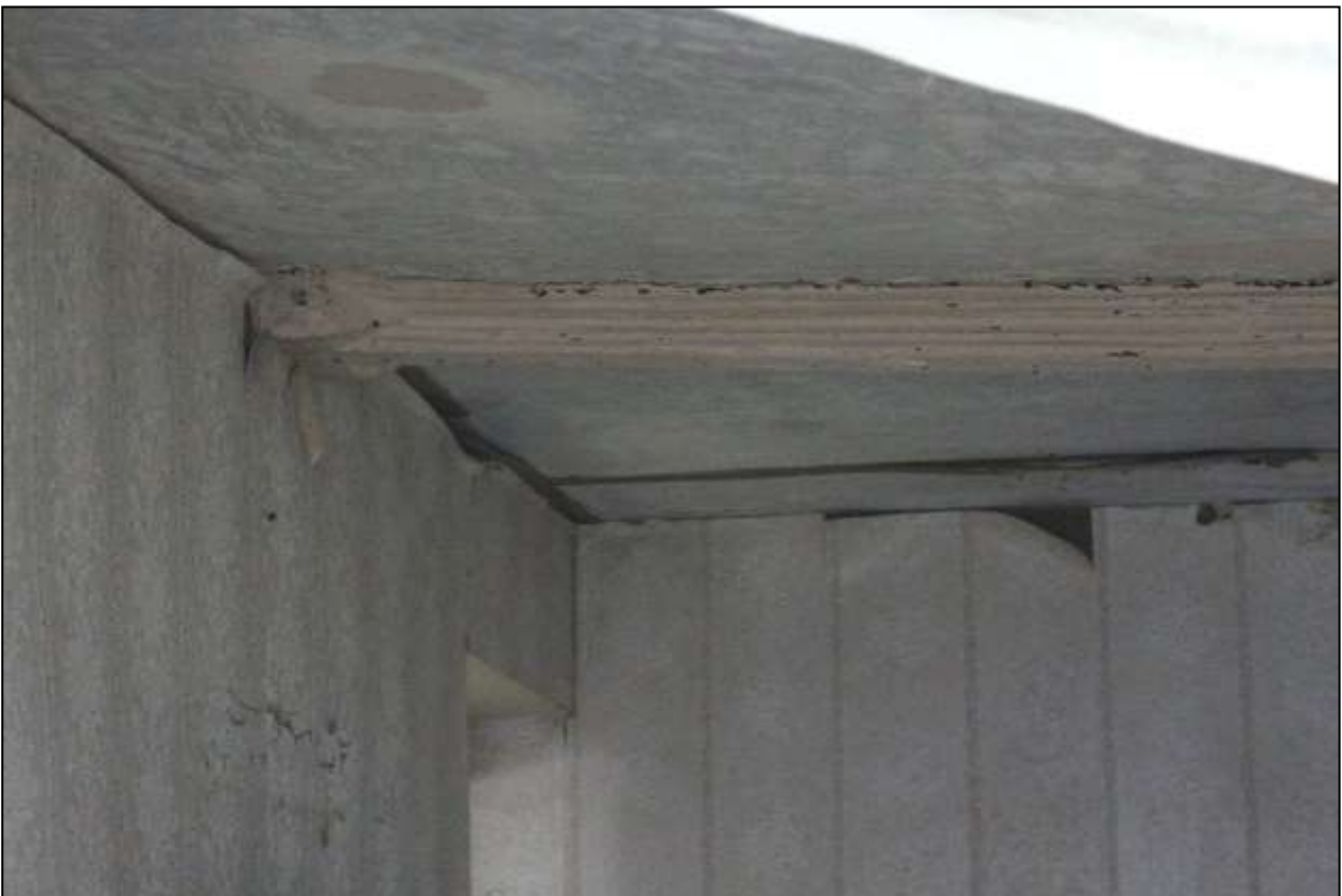
23. NORTHERN AXIAL BEAM IN R3; NOTE MOULDINGS ON SOUTH SIDE. VIEWED FROM THE SSE.
