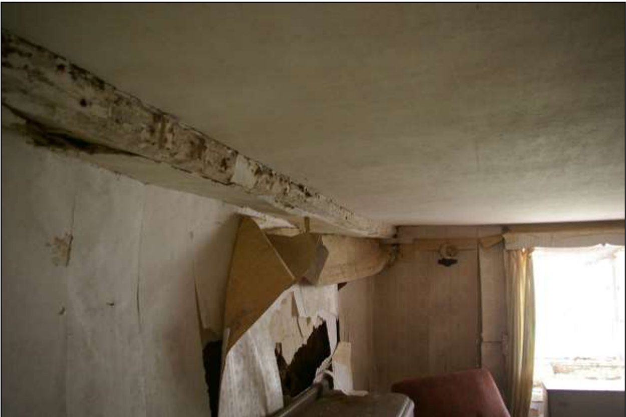
89. THE NORTH-EASTERN COB WALL OF R4 WITH CHAMFERED CEILING BEAM ABOVE; VIEWED FROM THE NORTH-WEST.
