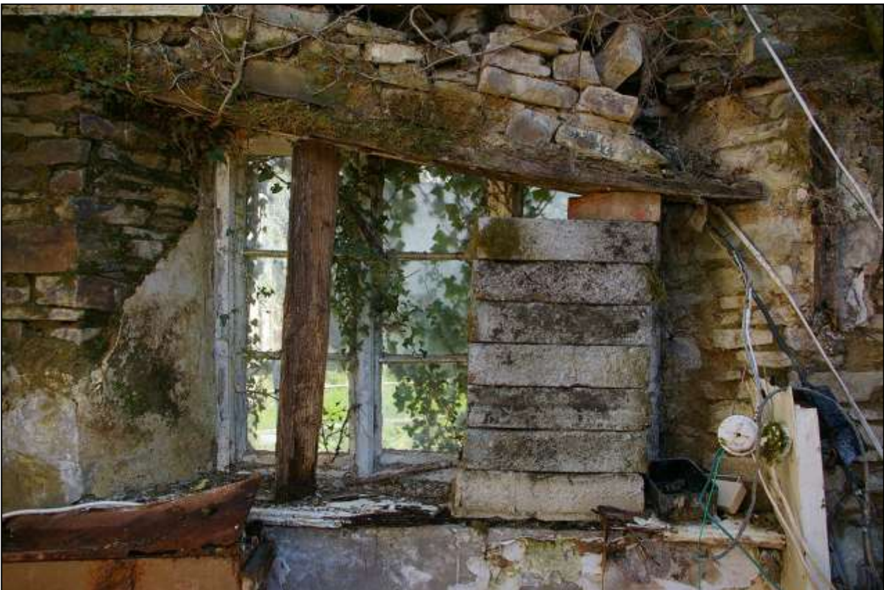
67. DETAIL OF THE GROUND FLOOR WINDOW IN R2 (W2), SOUTH WALL, SHOWING THREE-LIGHT 19 TH CENTURY CASEMENT WITH CHAMFERED MULLIONS, WIDE SPLAYED REVEALS AND TIMBER LINTEL. VIEWED FROM THE NORTH-WEST.
