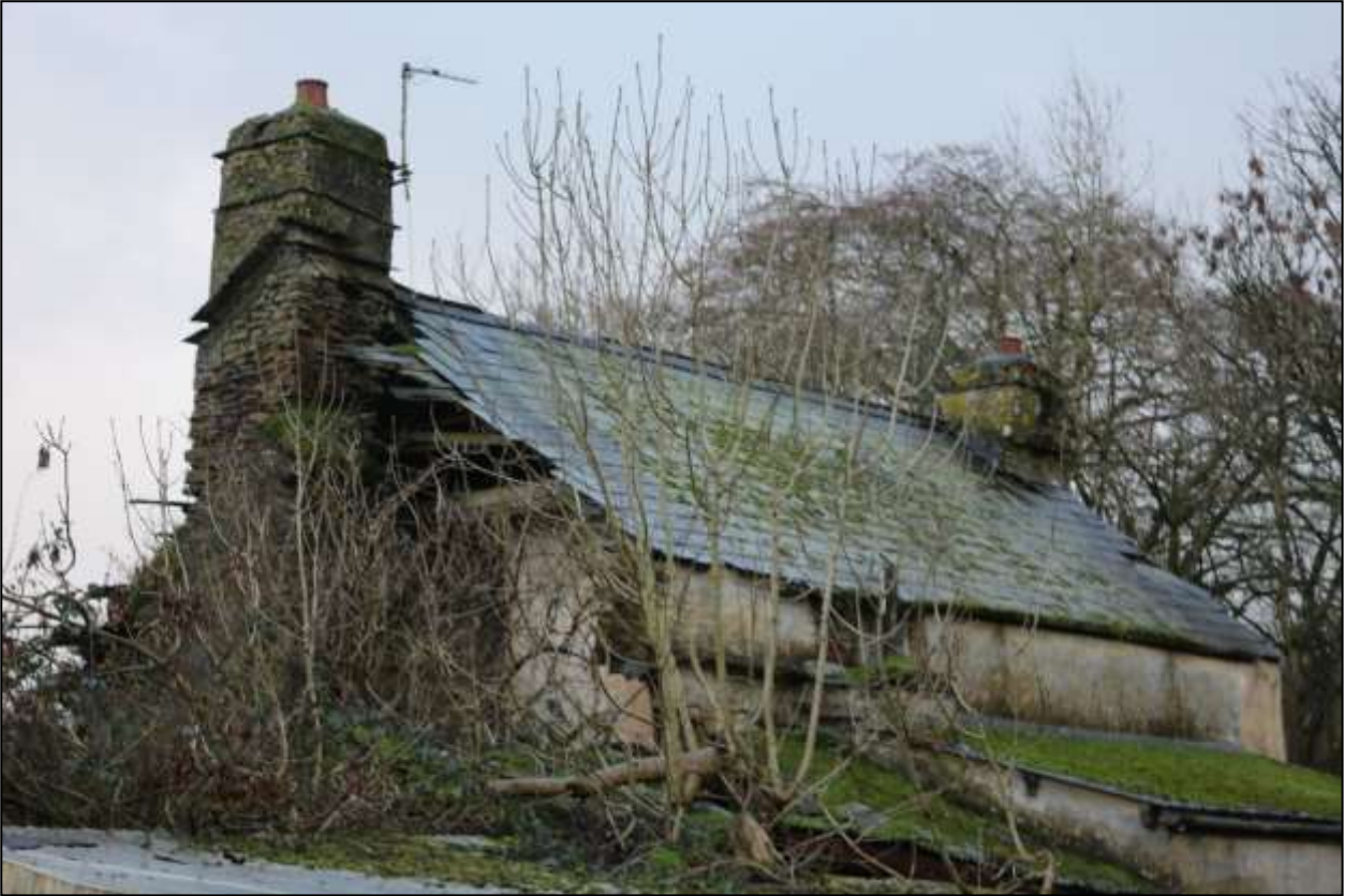
13. GENERAL VIEW OF REAR OF ROOFED FARMHOUSE ELEMENT; VIEWED FROM THE NORTH-EAST.
