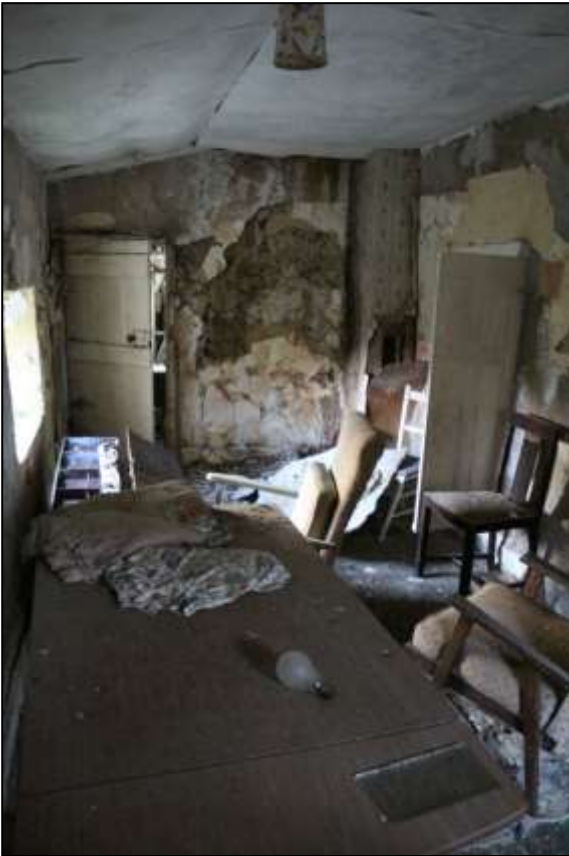
24. LEAN-TO R5 WITH DOOR (D9) TO R6 AT FAR LEFT; NOTE COB IN WALL FACE WHERE PLASTER HAS FALLEN AWAY; VIEWED FROM THE SOUTH-WEST.
