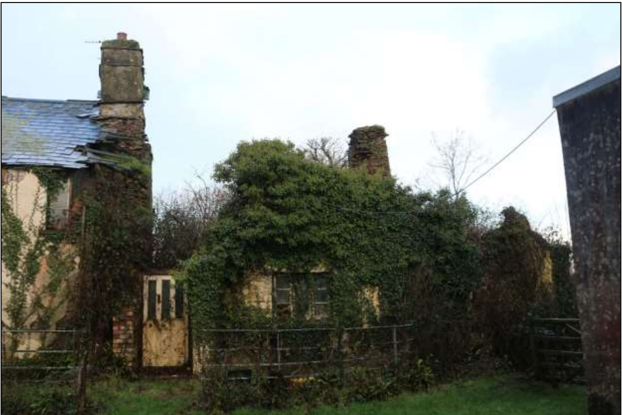
4. SOUTH-EAST ELEVATION OF COLLAPSED PART OF HOUSE, WITH SOUTH WINDOW OF R2 TO RIGHT OF FRONT DOOR. EASTERN AXIAL STACK VISIBLE BEHIND IVY, AND REMAINS OF COB WALLS OF R1 TO RIGHT. VIEWED FROM THE SSE.
