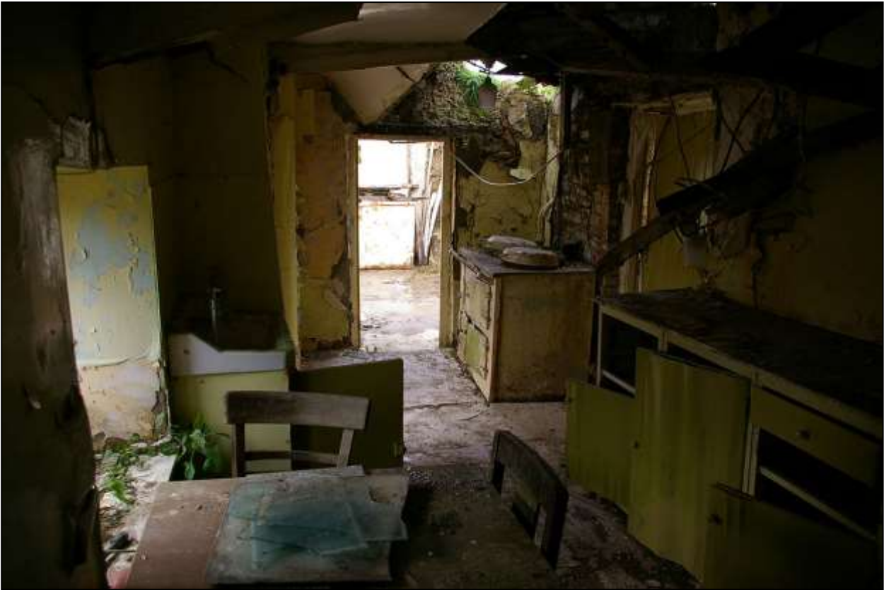
104.R6, ANOTHER EXTENSION TO THE FARMHOUSE, BEING A SCULLERY/KITCHEN; VIEWED FROM THE SOUTH-WEST.
