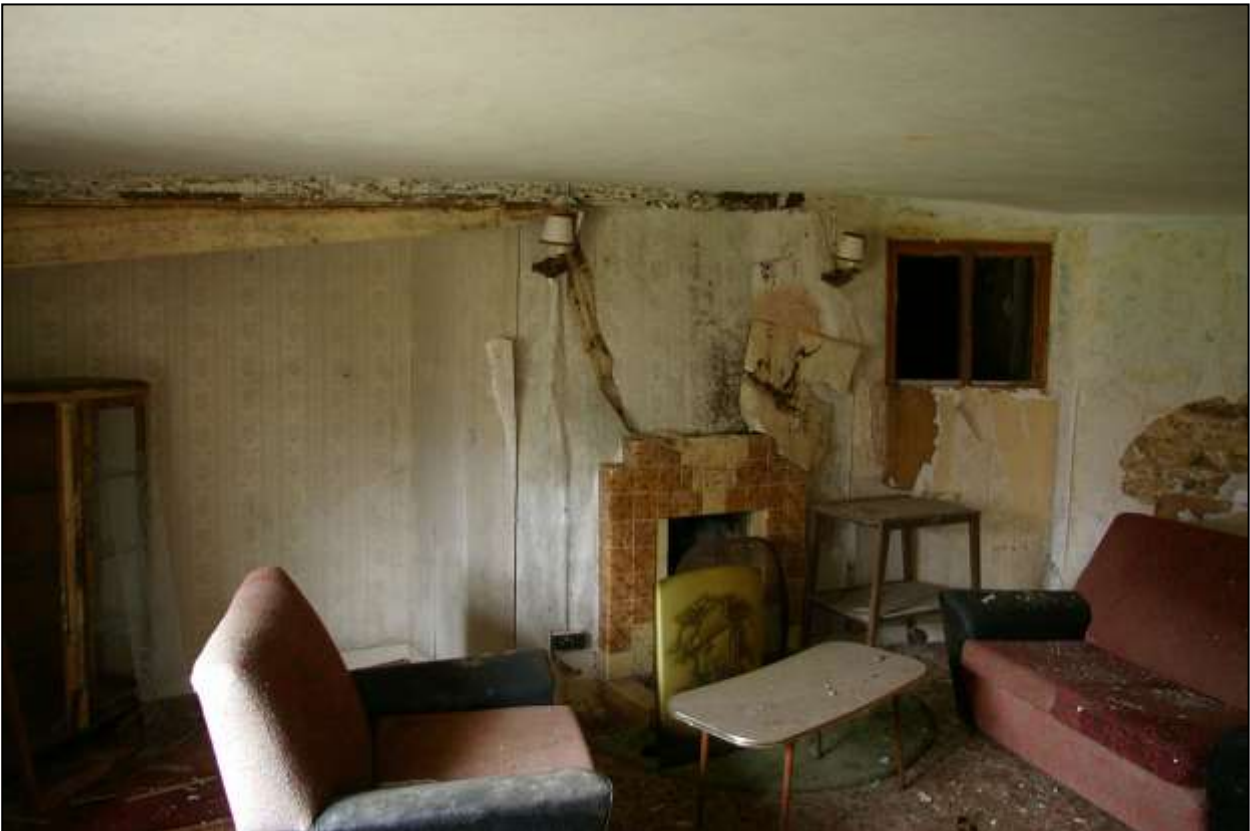
95. WEST WALL OF R4 WITH OFFSET STACK AND CUPBOARD TO RIGHT FRONTING FORMER WINDER STAIR; VIEWED FROM THE ENE.
