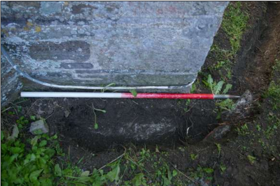
FIGURE 3: AREA 06, NORTH END SHOWING BUTTRESS FOUNDATIONS AND WALL {608} TO THE RIGHT OF THE SHOT; VIEWED FROM THE NORTH-WEST (1M SCALE).
