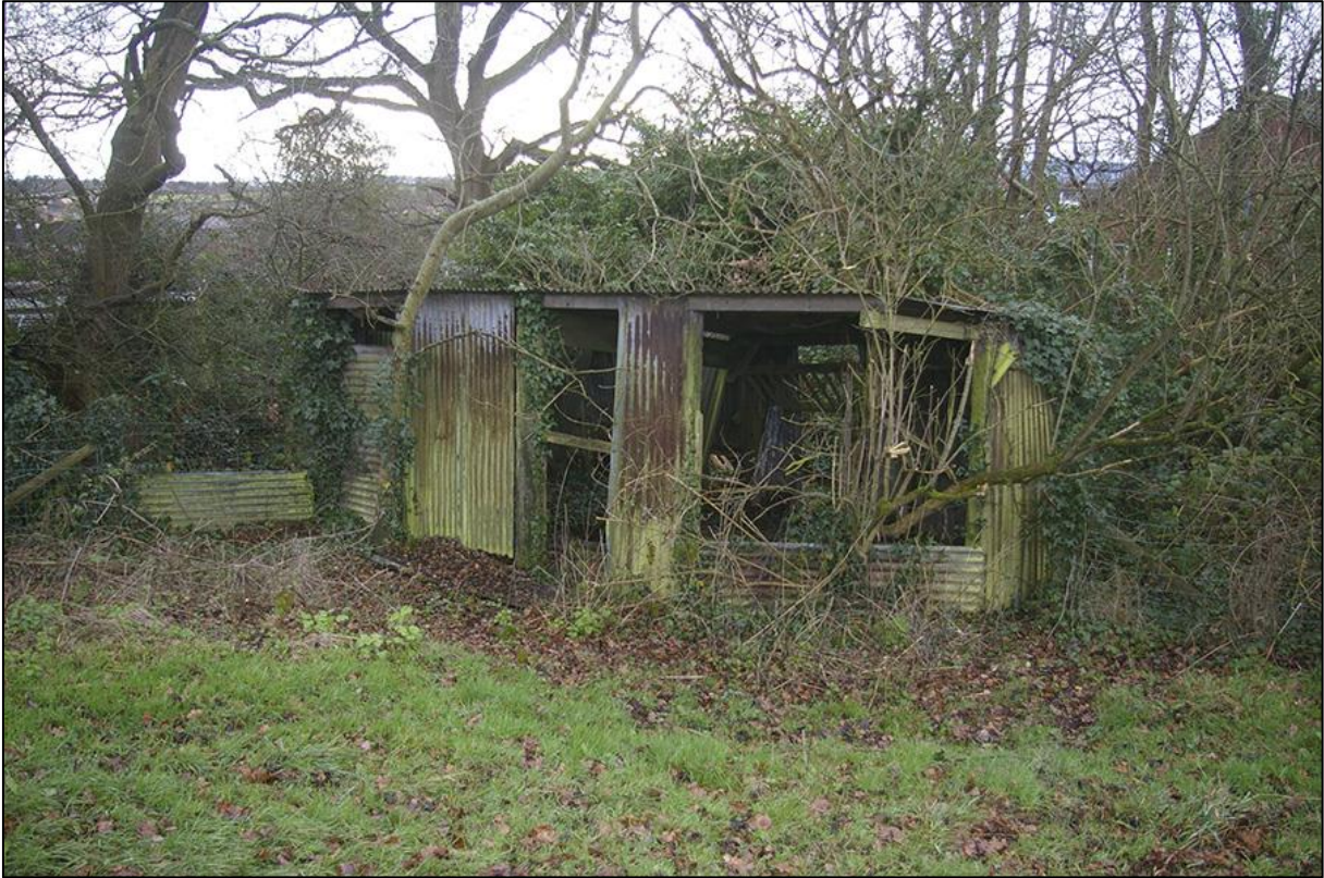
11. THE CORRUGATED SHED IN THE SOUTH CORNER OF THE SITE; VIEWED FROM THE NORTH (NO SCALE).
