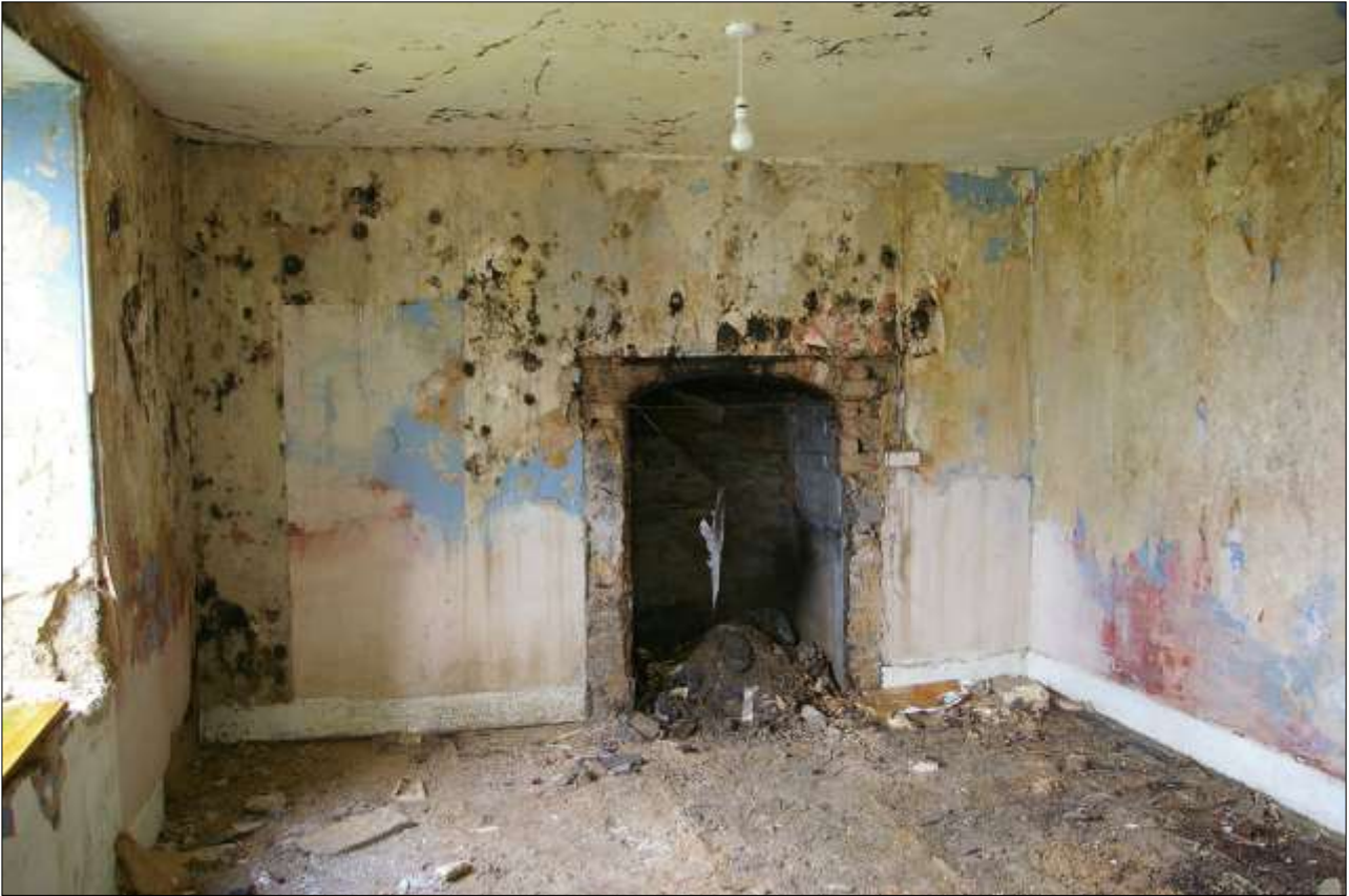
54. THE EAST END OF THE ROOM 6, WITH TALL SHALLOW BASKET ARCHED OPEN HEARTH; FROM THE WEST, NORTH-WEST.
