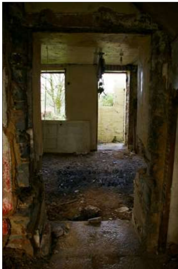
51. ROOM 2 ENTRANCE HALLWAY, LEADING INTO ROOM 6, THE REAR 19TH CENTURY EXTENSION; FROM THE SOUTH.
