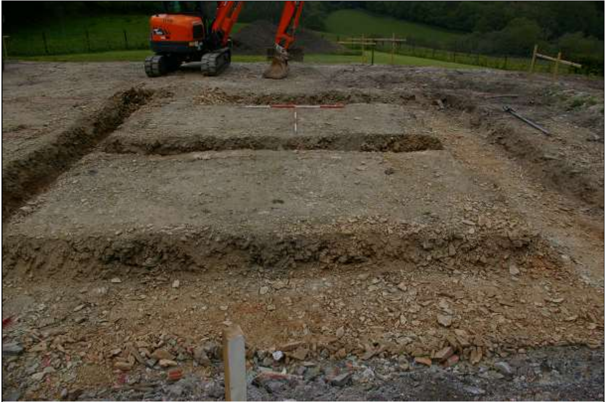
FIGURE 7: MONITORING THE NEW FOUNDATIONS OF THE HOUSE, WITH 2 X 2M SCALES; FROM THE EAST.
