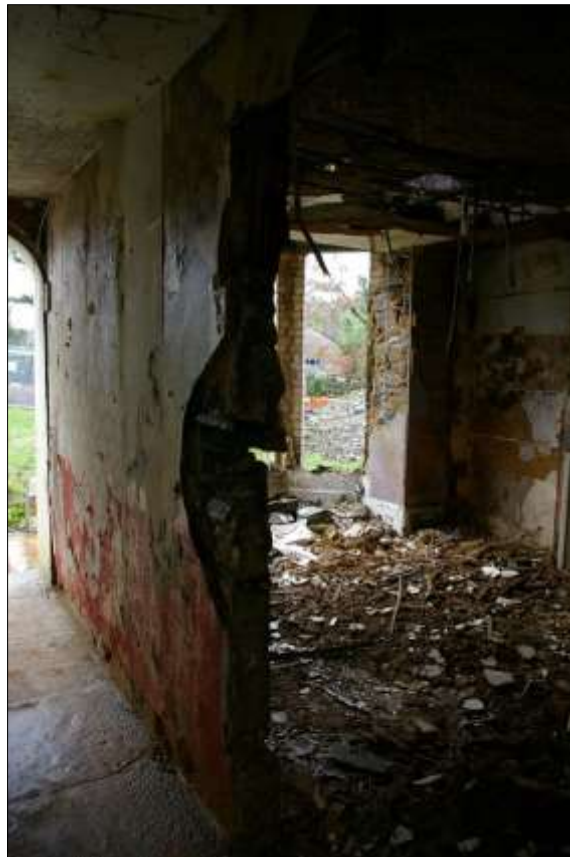
47. THE TIMBER FRAMED AND STONE RUBBLE NOGGIN PARTITION BETWEEN THE ENTRANCE HALLWAY AND ROOM 4; FROM THE NORTH-EAST.
