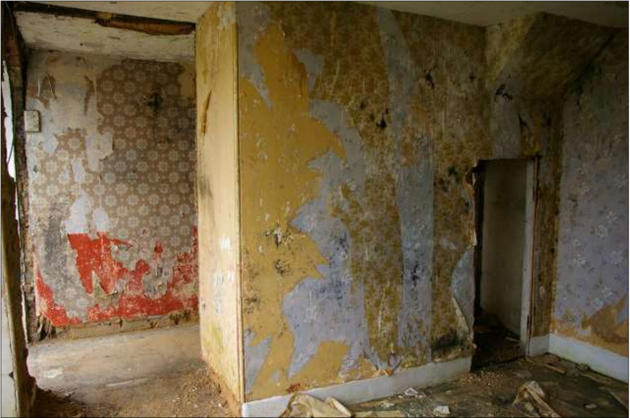
44. THE OPENING TO THE ENTRANCE HALLWAY FROM ROOM 3 AND THE EAST PARTITION WALL; FROM THE SOUTH-WEST..
