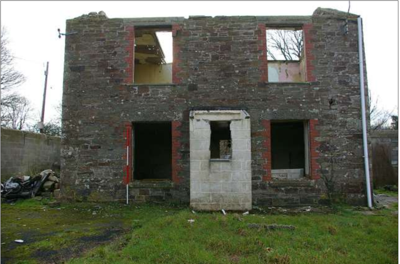
7. MORE DETAILED VIEW OF THE NORTH ELEVATION; FROM THE NORTH, 2M SCALE.
