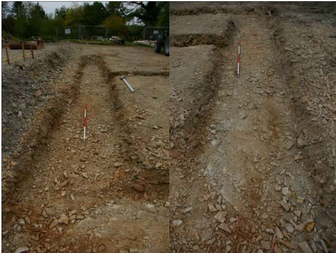
2. LEFT: THE EASTERN FOUNDATION TRENCH SHOWING DEGRADED BEDROCK; FROM THE SOUTH (2M SCALE).
