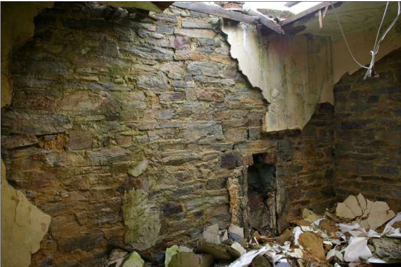
67. ROOM 8, THE EAST WALL AND SOUTH WALL. THE SMALL REDUCED OPENING IN THE EAST WALL IS AN ORIGINAL FIREPLACE WHICH HAS BEEN NARROWED FOR A LATER SMALLER GRATE; FROM THE NORTH-WEST.
