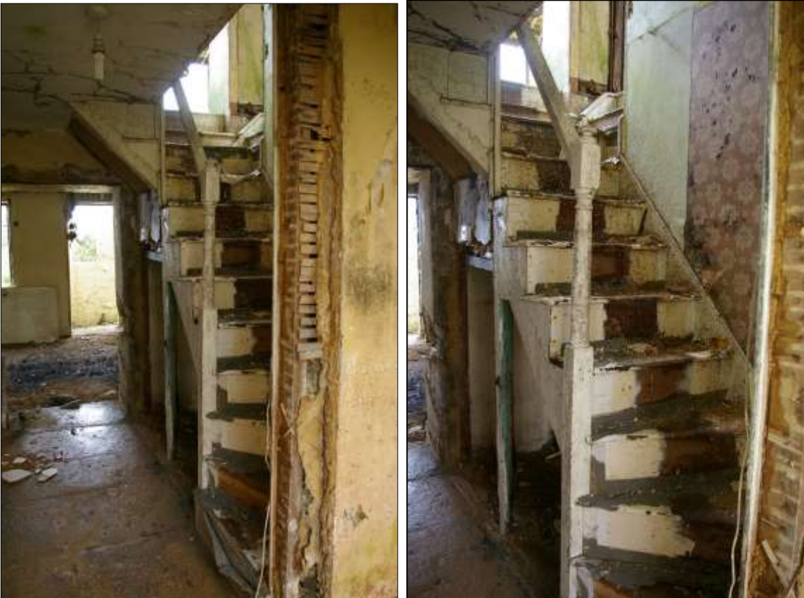
30. THE STAIRS, WITHIN AN L SHAPED PARTITION TO THE EAST OF THE ENTRANCE HALLWAY; FROM THE SOUTH, SOUTH-WEST. 31. RIGHT: THE STAIRS, POST FRAMED, OPEN STRING, WITH PILLARED NEWEL; FROM THE SOUTH-WEST.
