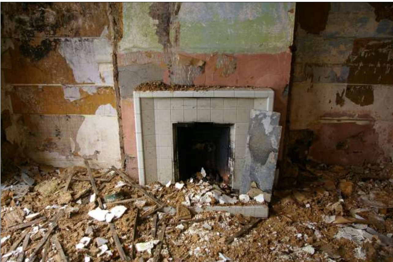
49. THE SHALLOW STACK IN THE PARLOUR, TILED MID-CENTURY, 1950S, SET INTO A BLOCKED OPEN HEARTH; FROM THE EAST.
