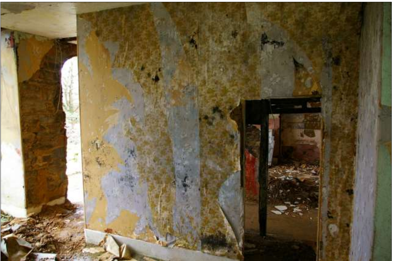
41. THE WEST PARTITION WALL OF ROOM 3, WHICH WRAPS AROUND THE STAIRS; FROM THE NORTH-EAST.
