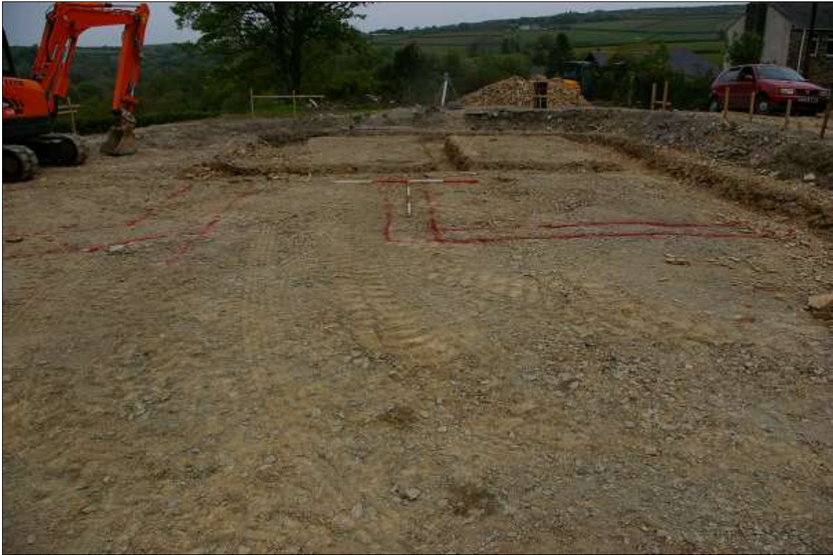
6. THE SITE FROM THE SOUTH, DURING MONITORING OF THE NEW FOUNDATION TRENCHES (2M SCALES).
