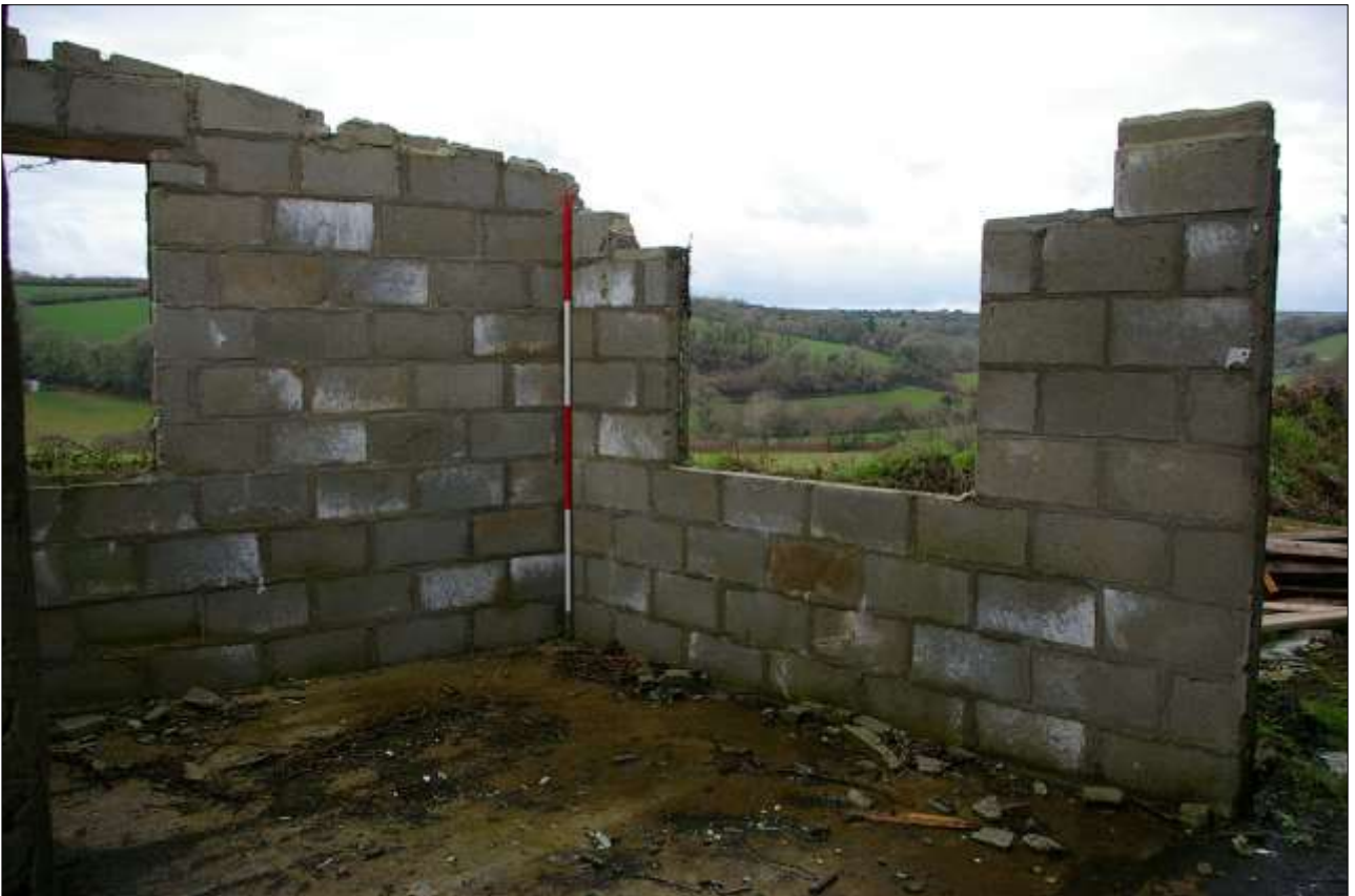
22. THE CONCRETE BLOCK EXTENSION, WITH WEST AND NORTH WALLS, 2M SCALE; FROM THE SOUTH-EAST.
