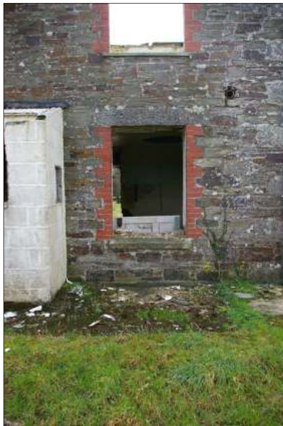
8. DETAIL OF W4 IN THE NORTH ELEVATION, SHOWING GRANITE LINTELS AND SILLS, WITH ADDITIONAL BRICK REVEALS, A LATER REPAIR; FROM THE NORTH.
