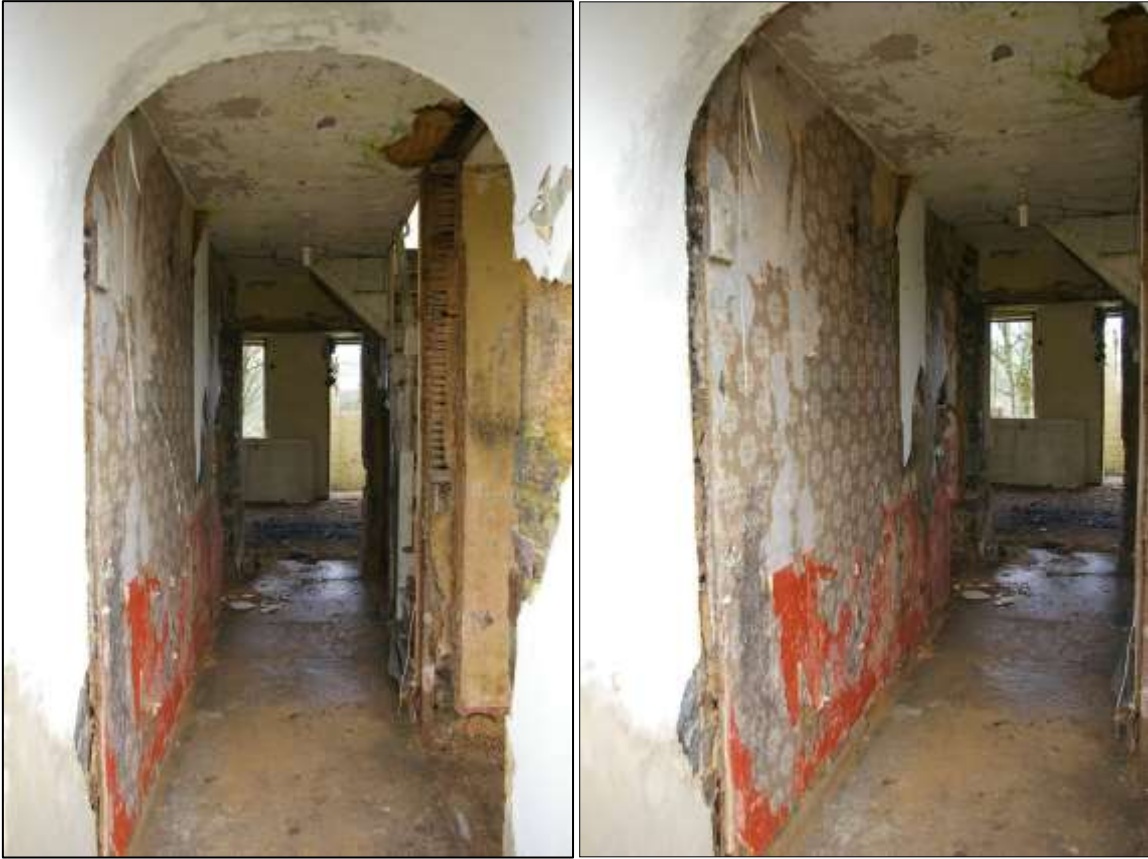
28. LEFT: VIEW INTO ROOM 2, THE ENTRANCE HALLWAY, WITH GRANITE SETS, TIMBER BRACED AND STONE NOGGIN PARTITION TO THE WEST, LATHE AND PLASTER PARTITIONS AROUND STAIR TO EAST; FROM THE SOUTH. 29. RIGHT: THE TIMBER FRAMED AND STONE RUBBLE NOGGIN PARTITION BETWEEN THE ENTRANCE HALLWAY AND THE PARLOUR; FROM THE SOUTH, SOUTH-EAST.
