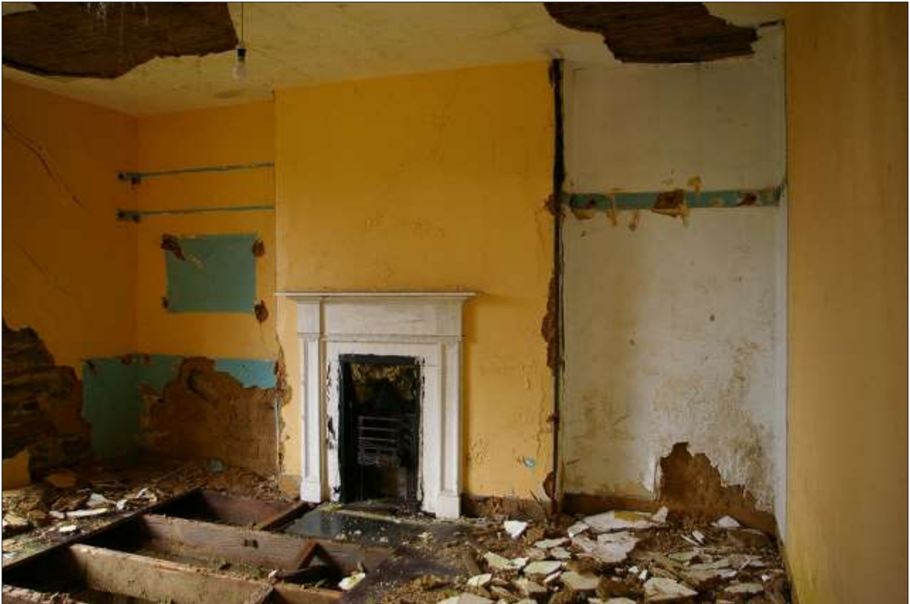
70. ROOM 10, THE SHALLOW STACK ON THE WEST WALL, WITH FINE LATE GEORGIAN OR EARLY 1800S, CAST IRON FOLIATE MOULDED HOB GRATE, TWO SHALLOW ALCOVES, SHELVES TO SOUTH, SCAR FROM ROW OF CLOTHING HOOKS TO NORTH; FROM THE EAST, NORTH-EAST.
