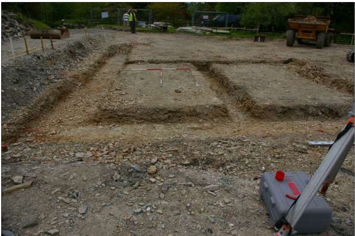
5. THE SITE, DURING THE MONITORING OF THE TRENCHES; FROM THE NORTH (2M SCALES).
