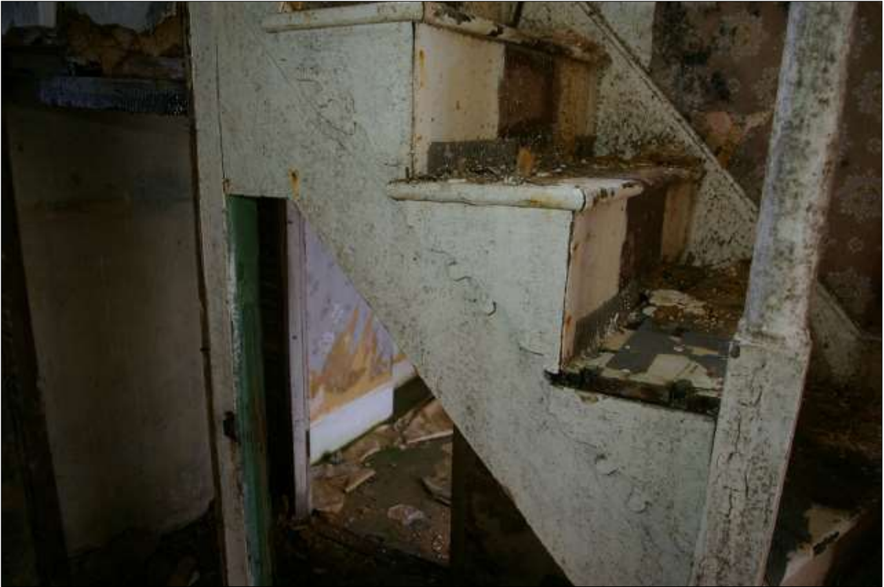
35. THE OGEE AND BEADED SCROLLWORK DETAILING TO THE OPEN STRING OF THE STAIRS; FROM THE WEST, SOUTH-WEST.
