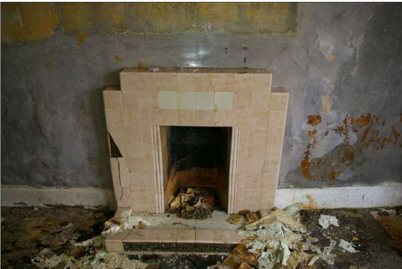
43. THE SMALL MID-20TH CENTURY, C.1950S FIREPLACE WHICH IS INSET INTO THE BLOCKED LARGE HEARTH TO THE KITCHEN, ROOM 3; FROM THE WEST.
