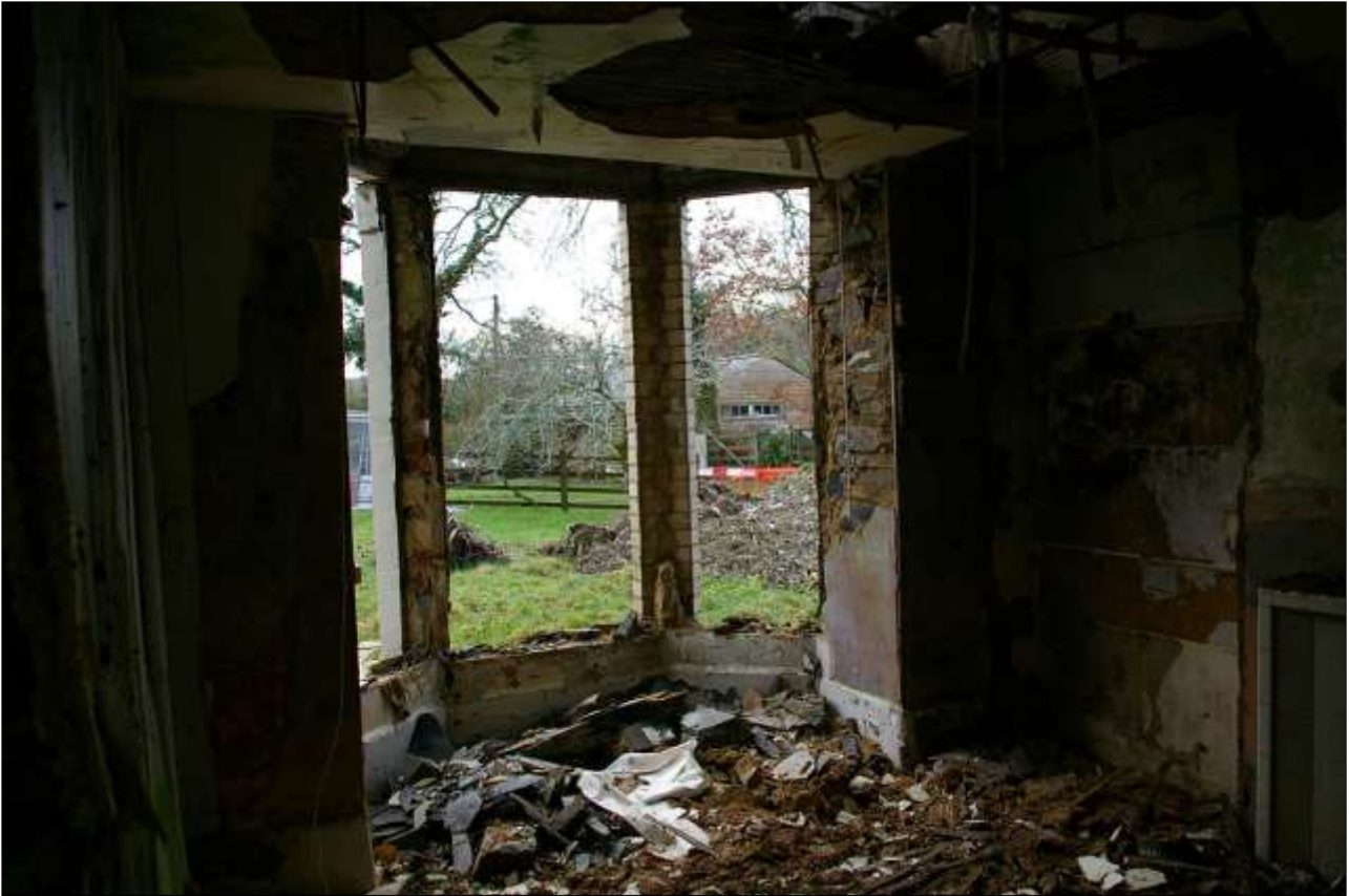
48. ROOM 4, THE PARLOUR, THE ADDED BRICK BAY WINDOW TO THE SOUTH WALL; FROM THE NORTH-EAST.
