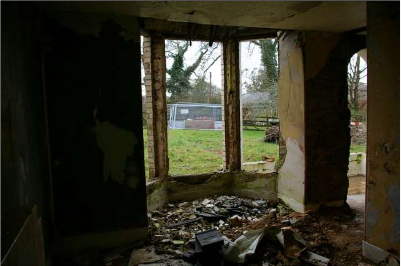
42. THE SOUTH WALL OF ROOM 3, THE ADDED BAY WINDOW; FROM THE NORTH-EAST.
