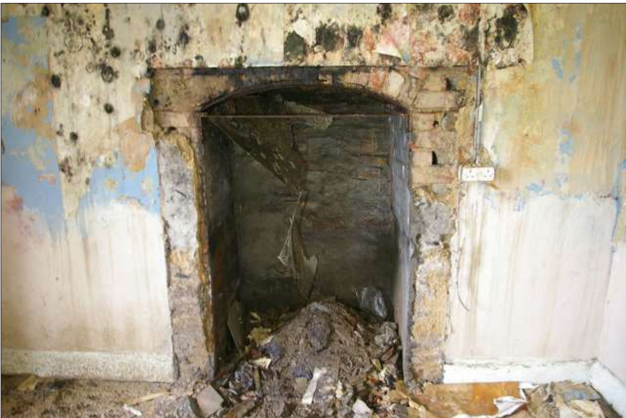
55. THE BRICK LINED SHALLOW BASKET ARCHED FIREPLACE, WITH IRON ARCHED BAR LINTEL, IRON FRAMING AND COLLAPSED REGISTER PLATE; FROM THE WEST.
