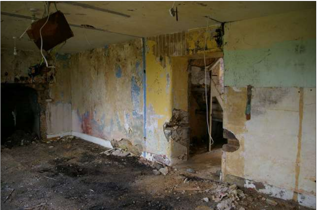
53. ROOM 6, THE 19TH CENTURY EXTENSION, LARGE OPEN SPACE, PARTITION WALLS REMOVED; FROM THE NORTH-WEST.
