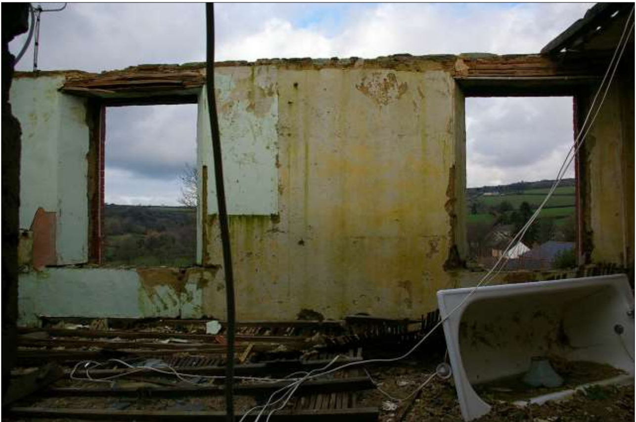
74. THE NORTH WALL OF ROOM 11, WITH TWO FIRST FLOOR WINDOWS AND SCARS OF PARTITIONS DIVIDING THE SPACE; FROM THE SOUTH.
