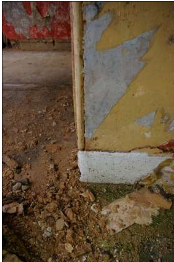
45. THE BEAD MOULDING ON THE CORNER WITH TALL FLAT PLASTER SKIRTINGS; FROM THE EAST.
