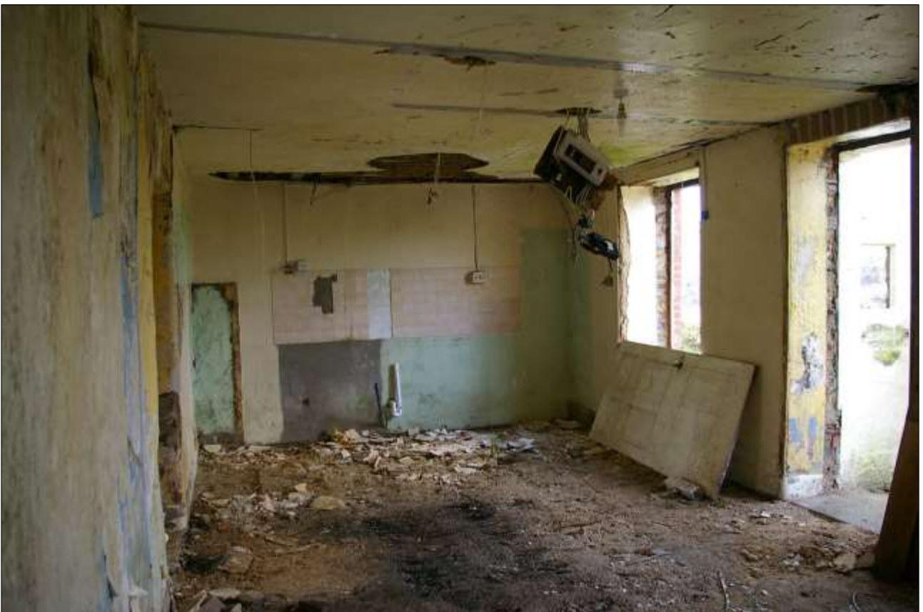
57. ROOM 6 FROM THE SOUTH-EAST, WITH TILED KITCHEN REMAINS VISIBLE ON THE WEST WALL.
