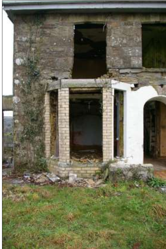
23. DETAIL OF ONE OF THE BRICK BAY WINDOWS TO THE SOUTH ELEVATION, ADDED TO THE EARLIER HOUSE; FROM THE SOUTH.
