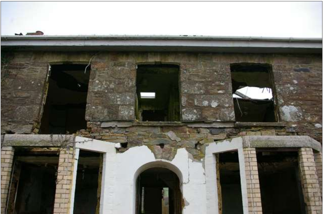
24. THE THREE ORIGINAL WINDOWS TO THE FIRST FLOOR OF THE SOUTH ELEVATION, SHOWING DRESSED STONE SEGMENTAL LINTELS, FROM THE SOUTH.
