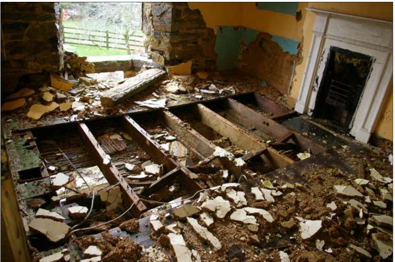
72. THE EVEN WIDTH WIDE BOARDED FLOOR, OVER NARROW BUT DEEP JOISTS, RUNNING NORTH-SOUTH, IN ROOM 10; FROM THE NORTH-EAST.
