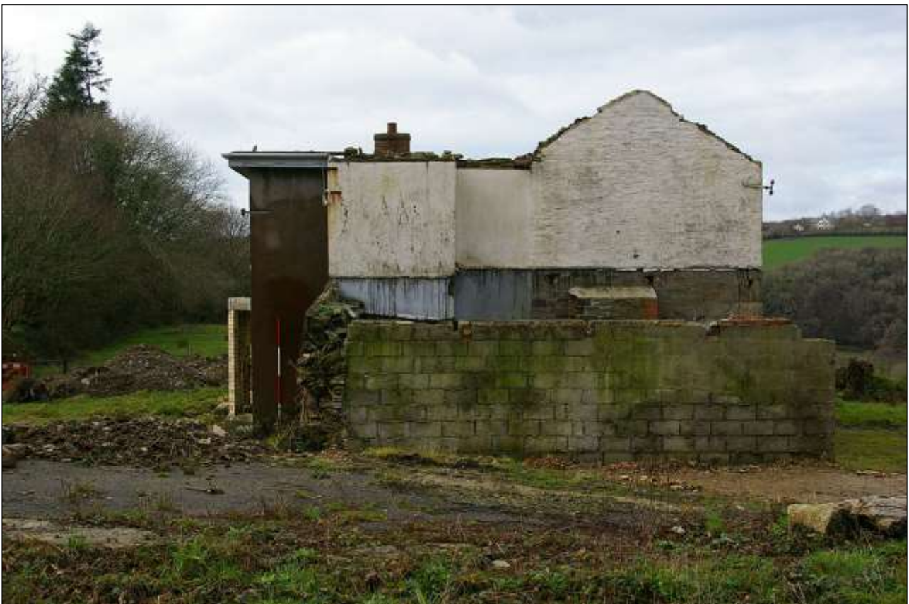
17. THE EAST ELEVATION OF THE HOUSE, WITH 2M SCALE; FROM THE EAST, SHOWING BOTH RANGES.
