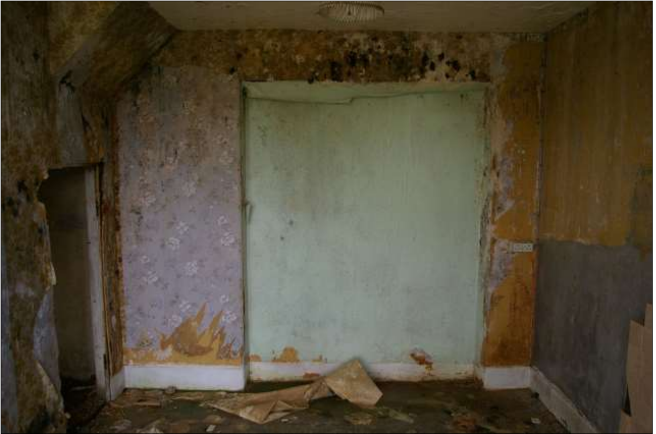
40. THE NORTH WALL OF ROOM 3, WITH LARGE BLOCKED RECTANGULAR OPENING, POSSIBLY A FORMER WINDOW; FROM THE SOUTH.
