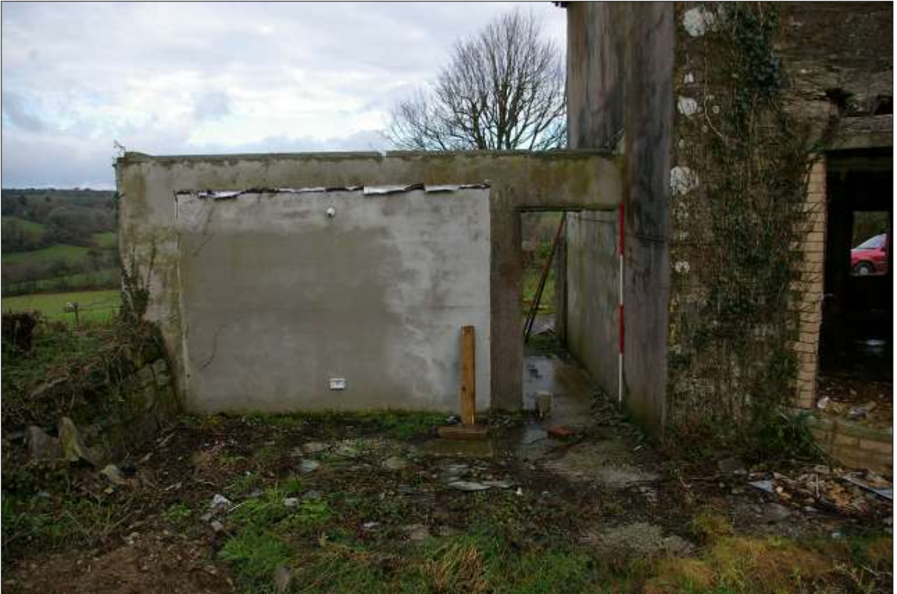
21. THE CONCRETE BLOCK EXTENSION TO THE WEST OF THE HOUSE, WITH 2M SCALE; FROM THE SOUTH.
