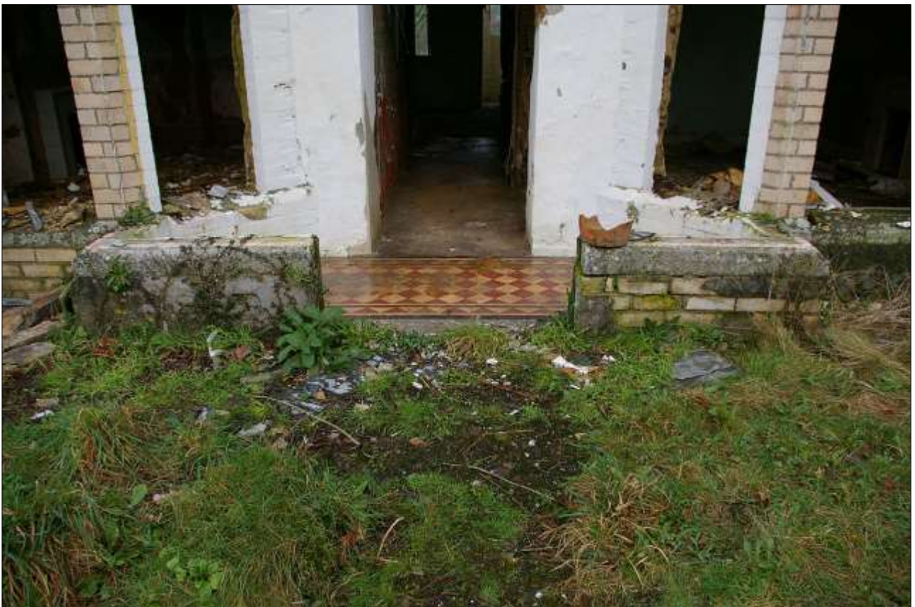
26. THE REMAINS OF THE FORMER FRONT PORCH, A 19TH CENTURY ADDITION, WITH GRANITE AND CERAMIC BRICK STRUCTURE, LIKE THE BAY WINDOWS; FROM THE SOUTH.
