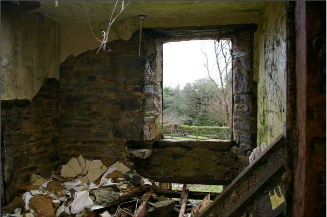
66. ROOM 8, THE SOUTH WALL, WITH INTERNAL TIMBER LINTEL AND OUTER STONE SEGMENTAL LINTEL; FROM THE NORTH.
