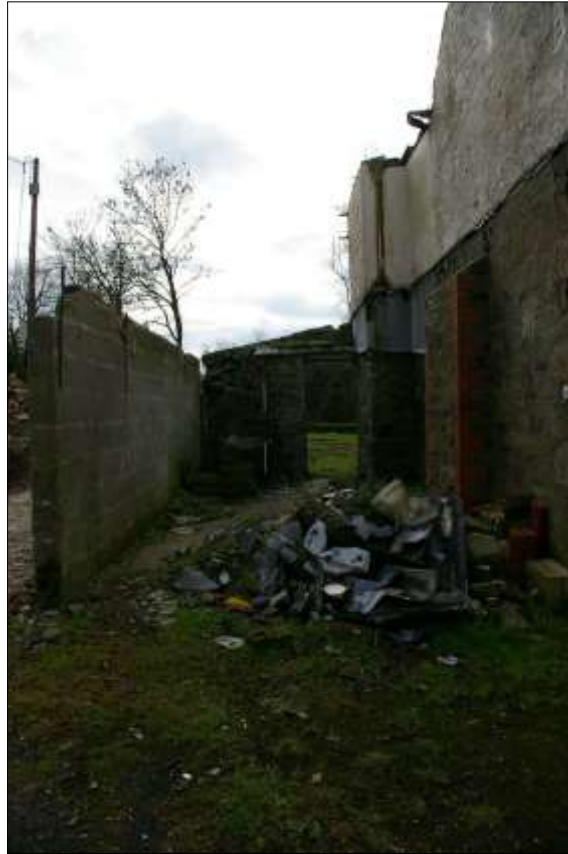
16. LEAN-TO ON THE EAST ELEVATION, STONE RUBBLE TO THE SOUTH END, CONCRETE BLOCK TO THE EAST WALL, CONCRETE FLOOR, 2M SCALE; FROM THE NORTH.
