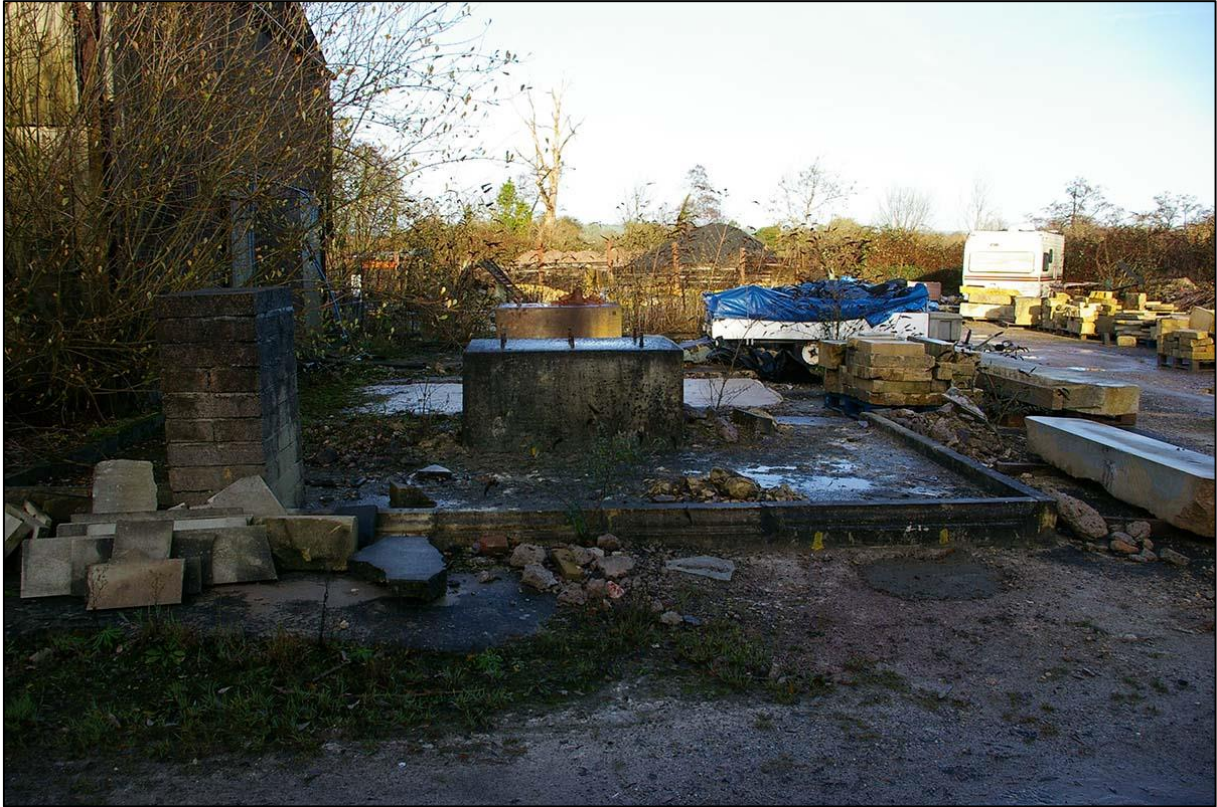
VIEW OF SOME OF THE CONCRETE PADS WITH FIXINGS FOR MACHINERY; VIEWED FROM THE SOUTH.
