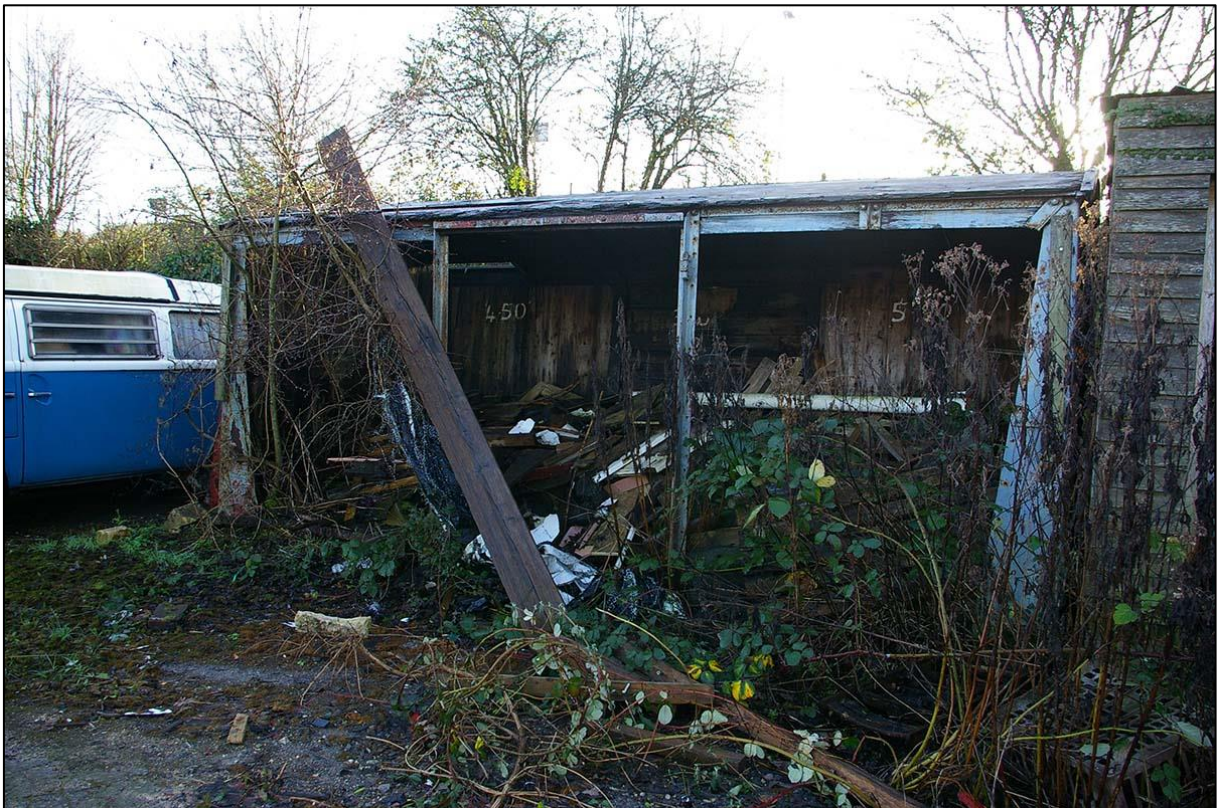
THE BEST PRESERVED OF THE FREIGHT CARRIAGES, WHICH HAS RETAINED ITS ROOF AND ITS HEAVY CORRUGATED ENDS; VIEWED FROM THE NORTH-WEST.
