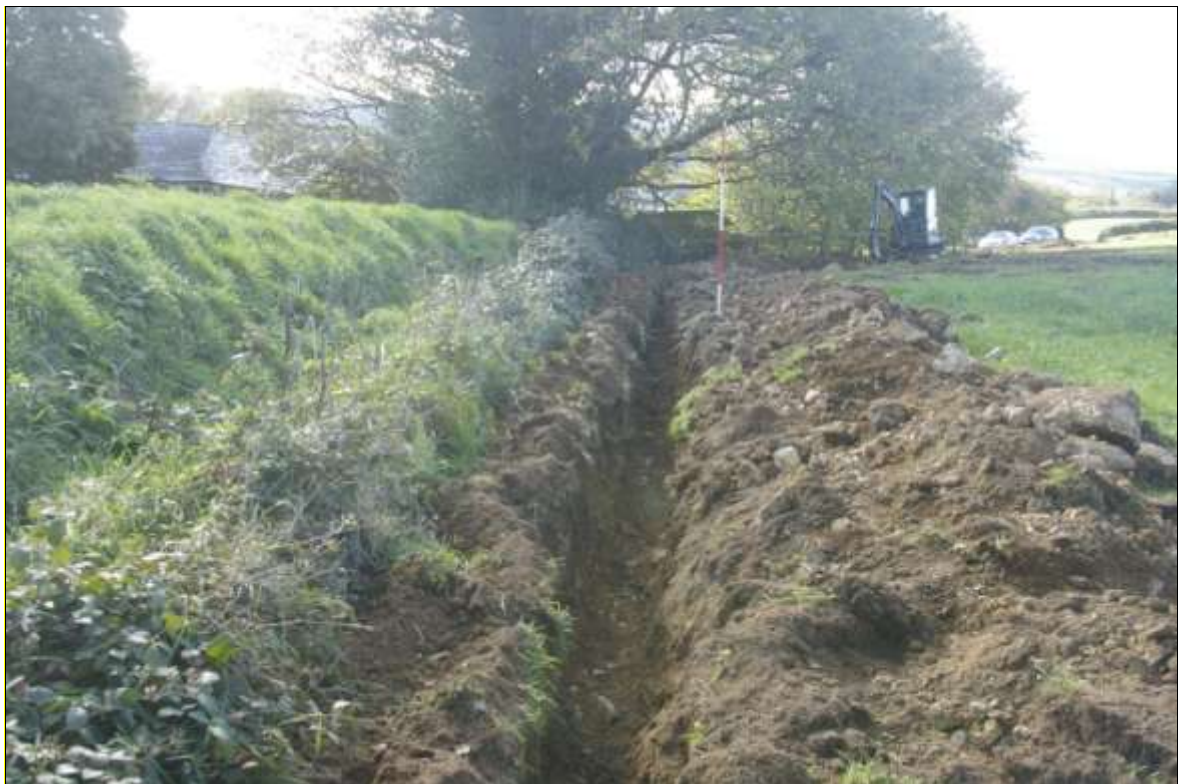
FIGURE 3: VIEW ALONG THE CABLE TRENCH SOUTH END; VIEWED FROM THE NORTH-EAST (2M SCALE).
