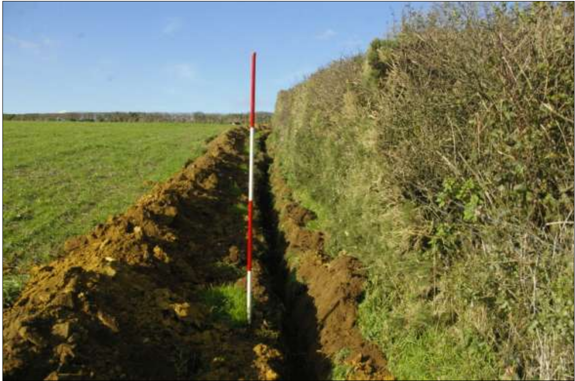
FIGURE 2: VIEW ALONG THE CABLE TRENCH NORTH END; VIEWED FROM THE SOUTH (2M SCALE).
