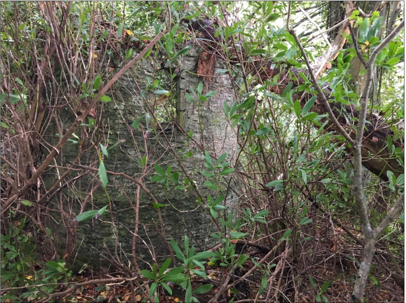
FOLLY SHOWING THE FALLEN TREE, RESTING ON THE STRUCTURE (COURTESY OF THE AGENT).
