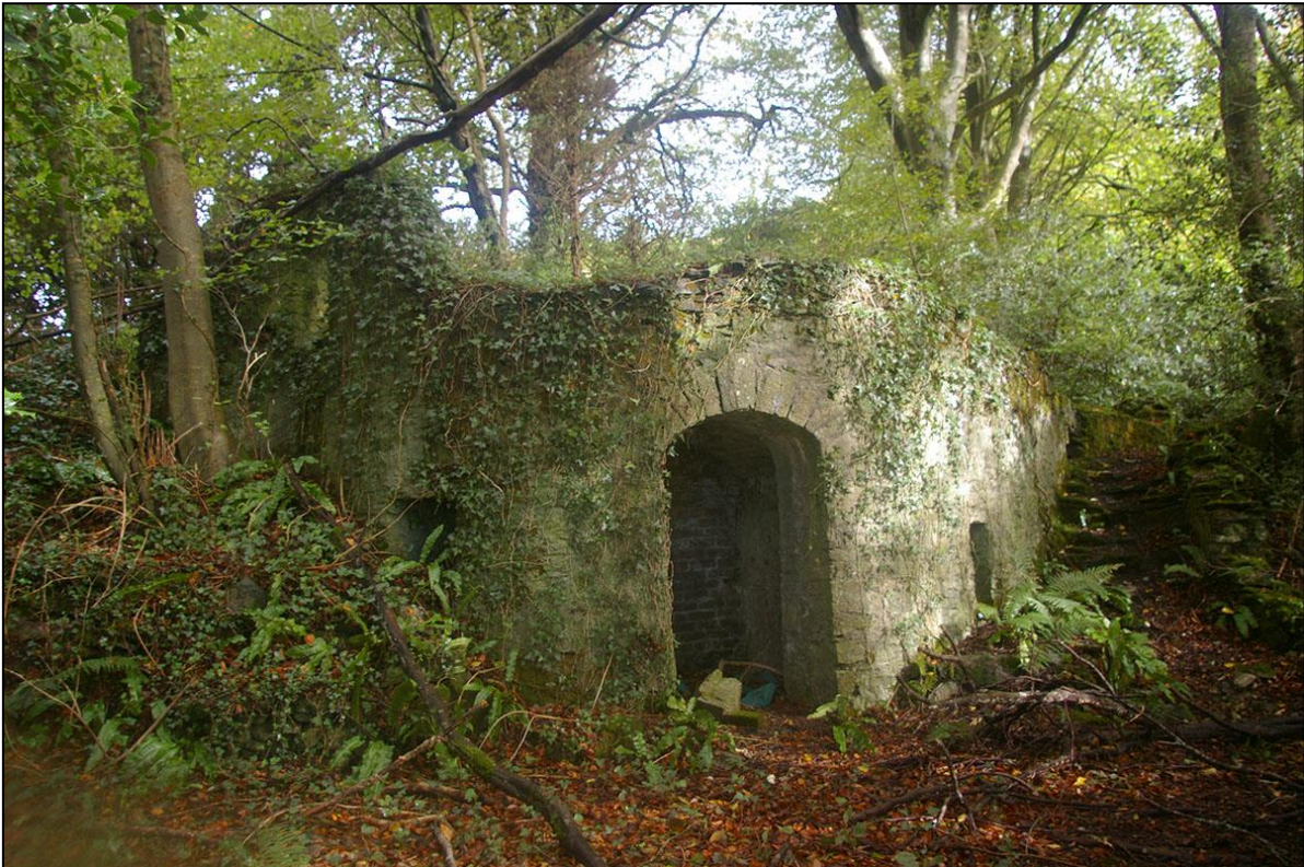
THE BRICK VAULTED SHELTER BUILT UNDER THE TERRACE TO THE WEST OF THE SUMMERHOUSE; FROM THE WEST-SOUTH-WEST.
