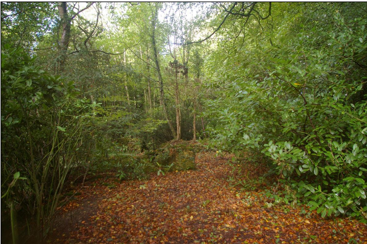
THE SOUTH-WEST WALK ON THE APPROACH TO THE SUMMERHOUSE AND TERRACE, SHOWING HOW IT IS BEING RECLAIMED BY NATURE, WITH MOSS, LEAVES AND DEBRIS OBSCURING THE STRUCTURE; FROM THE SOUTH-EAST.
