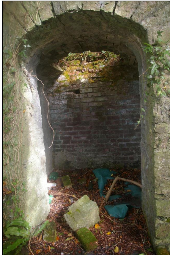
VIEW OF THE BRICK VAULTED ROOM UNDER THE TERRACE, PART OF THE CEILING OF WHICH HAS GIVEN WAY; FROM THE WEST.
