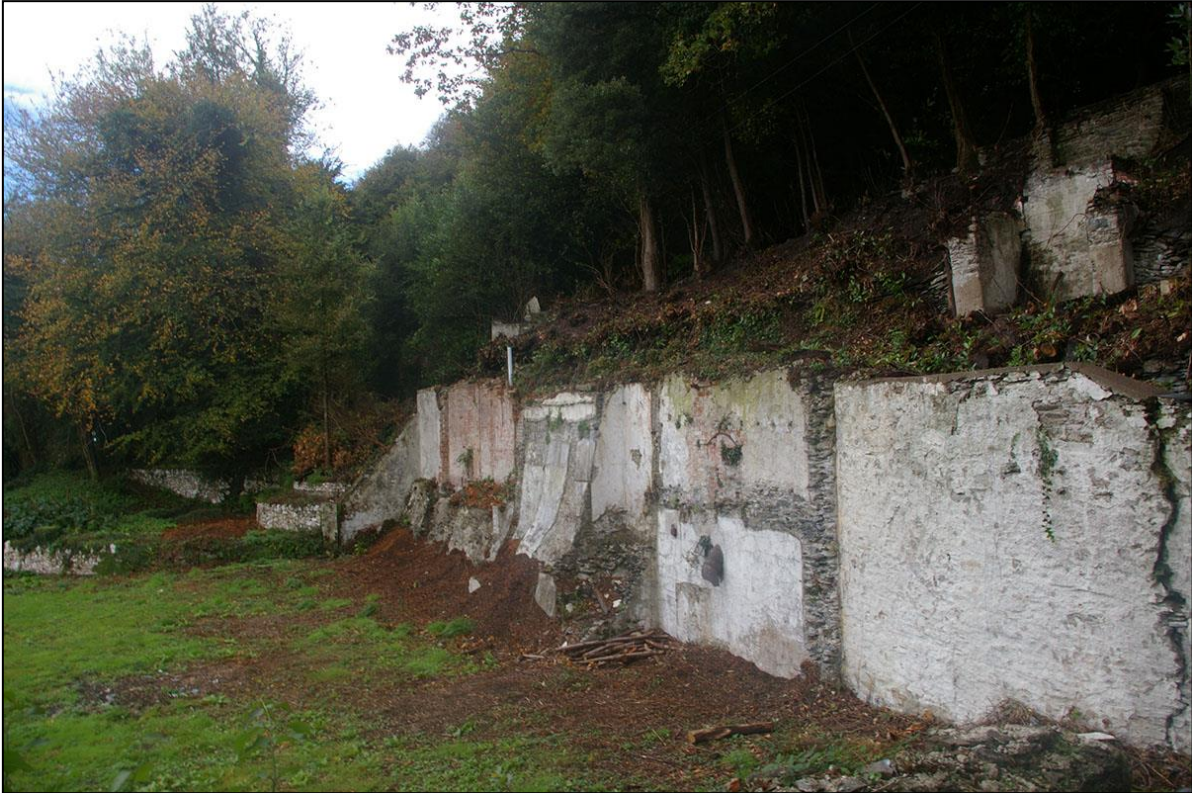
THE NORTH WALLS OF THE HOUSE AND RETAINING WALL TO THE REAR TERRACE; FROM THE EAST-SOUTH-EAST.
