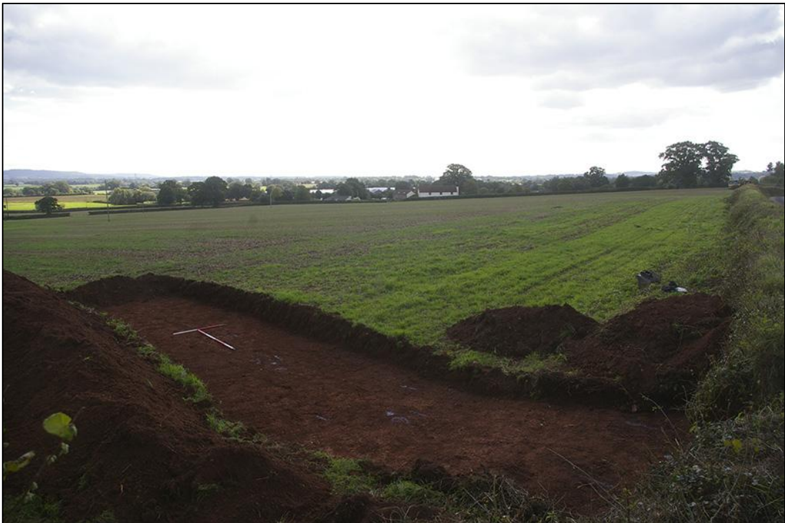
FIGURE 6: SOAK-AWAY 1 EXCAVATED TO THE DEPTH OF IN-SITU/WEATHERED NATURAL AND THE SITE; VIEWED FROM THE NORTH-WEST (1M AND 2M SCALE).
