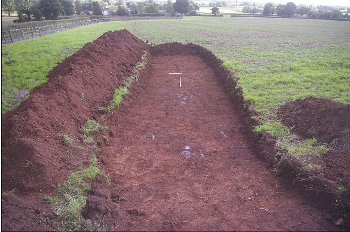
SOAK-AWAY 1 EXCAVATED TO THE DEPTH OF IN-SITU/WEATHERED NATURAL; VIEWED FROM THE WEST (1M AND 2M SCALE).
