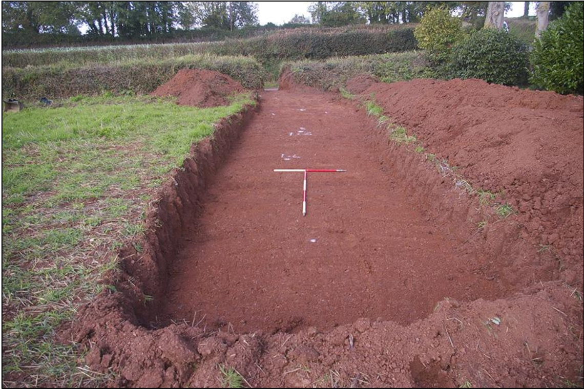
FIGURE 5: SOAK-AWAY 1 EXCAVATED TO THE DEPTH OF IN-SITU/WEATHERED NATURAL; VIEWED FROM THE EAST (1M AND 2M SCALE).
