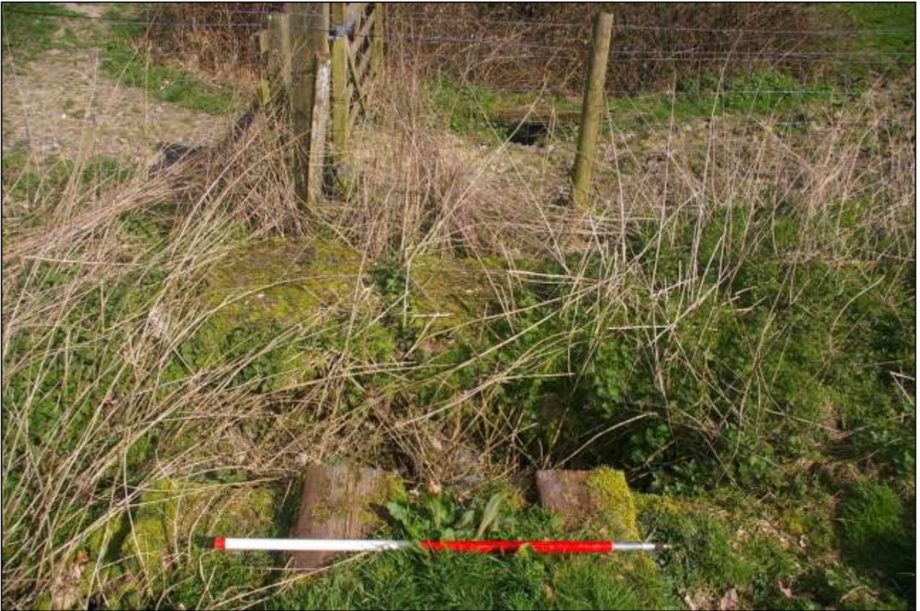
11. VIEW OF DRAIN TO THE SOUTH-EAST OF THE SITE RUNNING EAST; VIEWED FROM THE WEST (1M SCALE).
