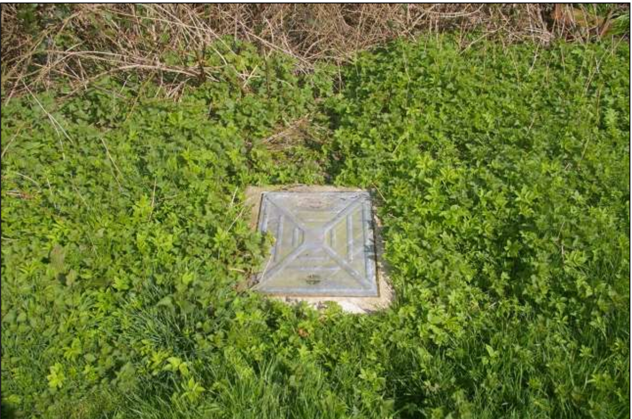
2. MANHOLE COVER SOUTH OF PAYNES COTTAGES; VIEWED FROM THE WEST (NO SCALE).
