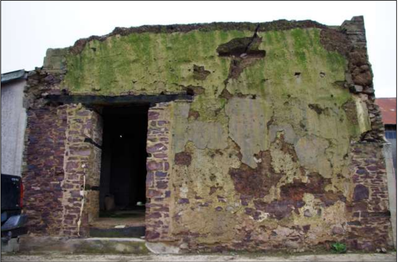
5. END WALL OF THE MEDIEVAL FORMER THRESHING BARN; VIEWED FROM THE SOUTH-SOUTH-EAST (NO SCALE).
