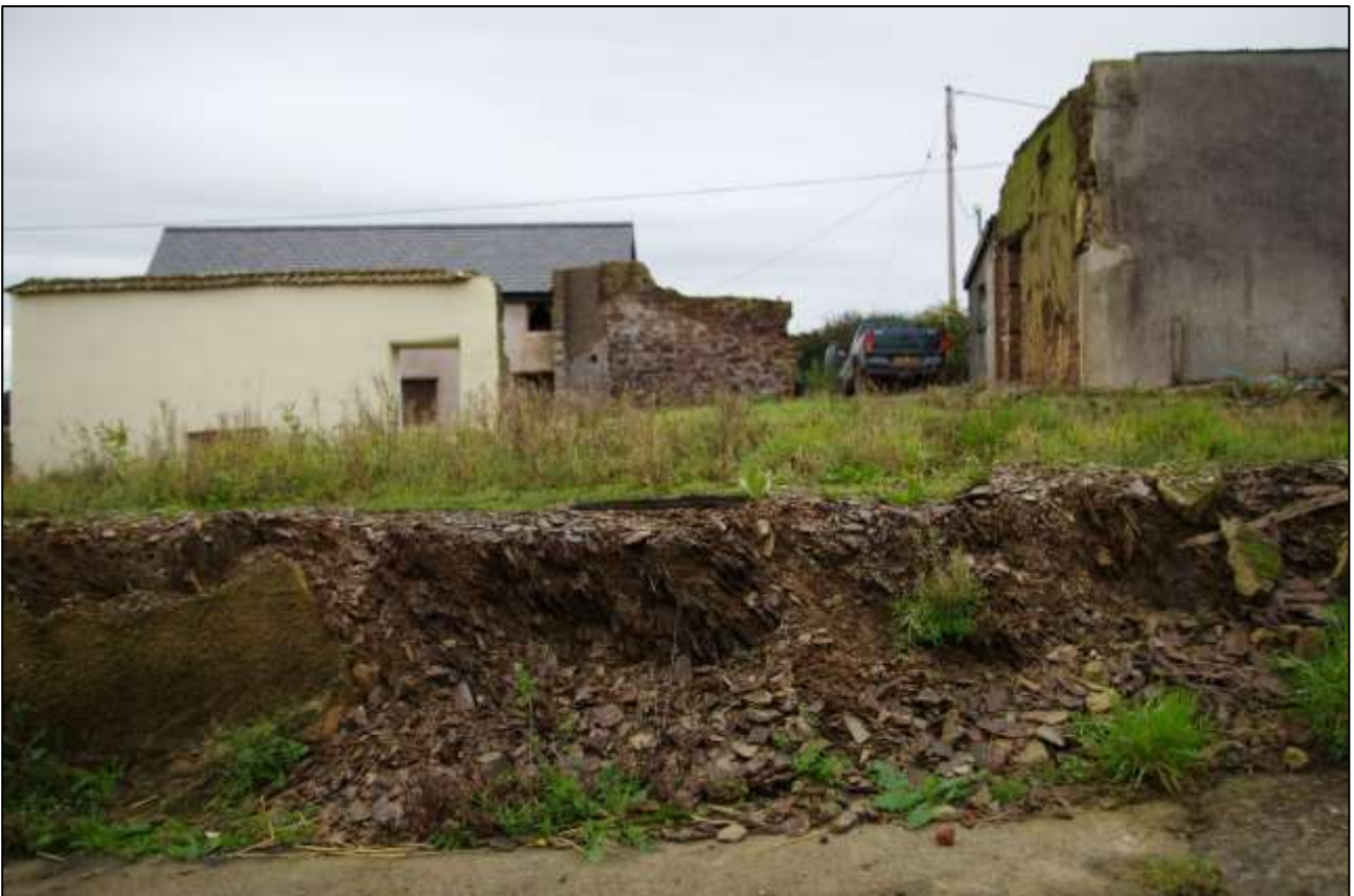
4. THE NORTH-EAST GABLE END OF THE FORMER HOUSE, SHOWING HOW THE COB WALLS OF THE BUILDING HAD BEEN PERCHED UP ON A STEP CUT INTO THE SHILLET BEDROCK; VIEWED FROM THE NORTH-EAST (NO SCALE).
