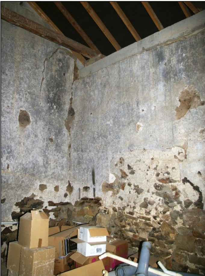
25. SOUTH-EAST CORNER OF BARN, FROM NORTH-WEST. NOTE BLOCKED DOOR IN SOUTH WALL AT LOWER RIGHT.
