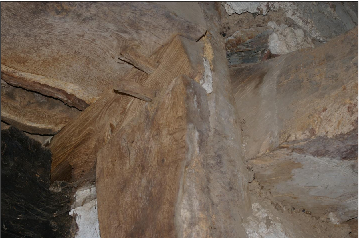
31. C18 RAISED LINTEL OVER WEST CHEEK OF THRESHING DOOR, ON CANTILEVERED SUPPORT FOR PENTICE ROOF, FACE-PEGGED TO CRUCK FOOT, SEEN VERTICALLY HERE AT MIDDLE RIGHT, WITH C18 INSERTED LOFT BEAM TO RIGHT. LOOKING UP FROM NORTH-EAST.
