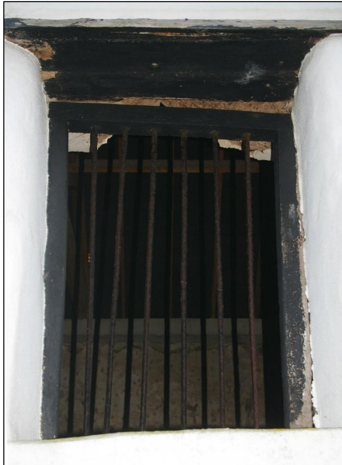
9. INSERTED C18 WINDOW IN SOUTH WALL OF CIDER BARN. VIEW FROM SOUTH.
