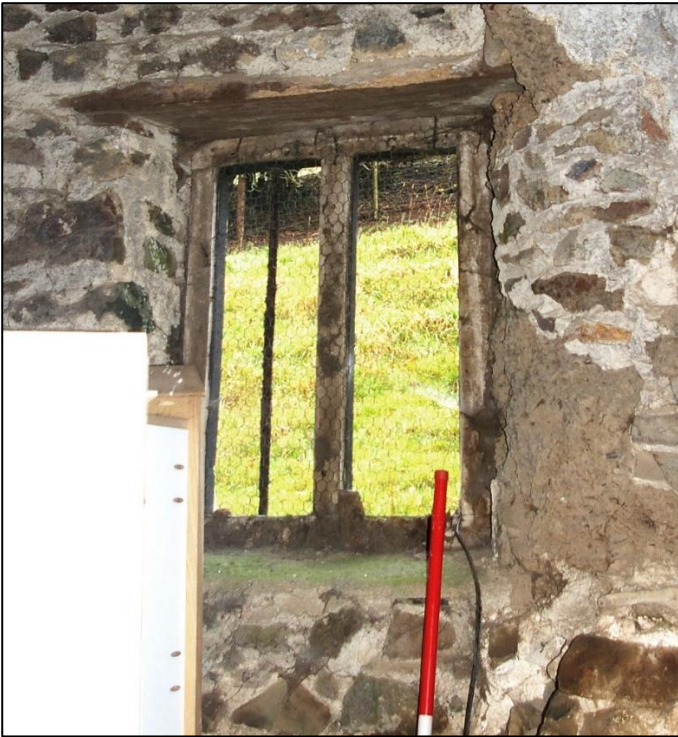
22. C18 WINDOW IN C19 RUBBLE FILL OF NORTH THRESHING DOOR. VIEW FROM SOUTH.
