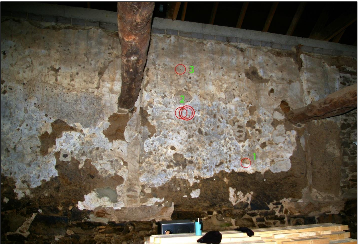
37. POSITIONS OF APOTROPAIC MARKS IN THIRD BAY FROM WEST ON NORTH WALL. VIEW FROM SOUTH. NOTE BLOCKED SOCKETS OF PROBABLE STAIR LADDER ABOVE AND TO RIGHT OF MARK 1.
