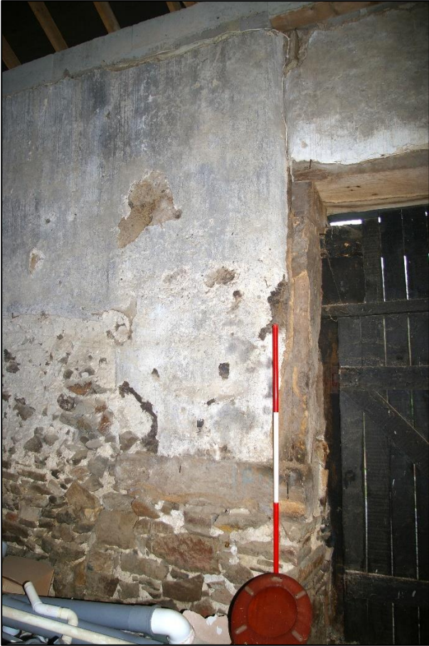
26. EAST JAMB OF THRESHING DOOR IN SOUTH WALL, FROM NORTH-WEST. NOTE BLOCKED DOOR TO LEFT AND INSET WALL FACE OVER LINTEL.
