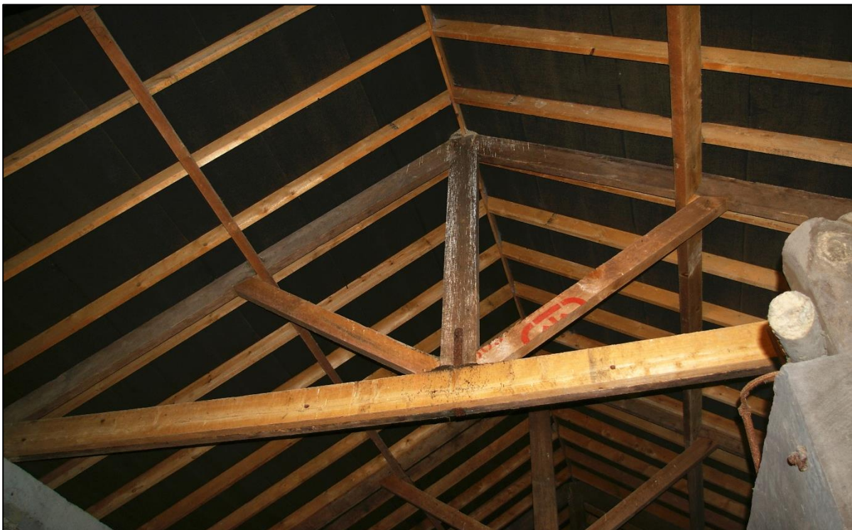
35. LATER C19 ROOF TRUSS WITH LATE C20 REPAIRS (IN PALER WOOD), LOOKING UP FROM EAST END OF BARN.
