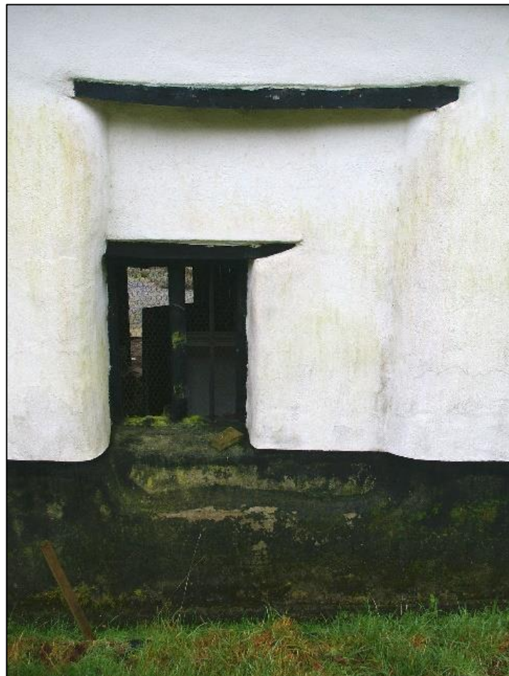
6. DRAUGHT DOOR AT REAR OF CIDER BARN, BLOCKED IN C19. VIEW FROM NORTH.
