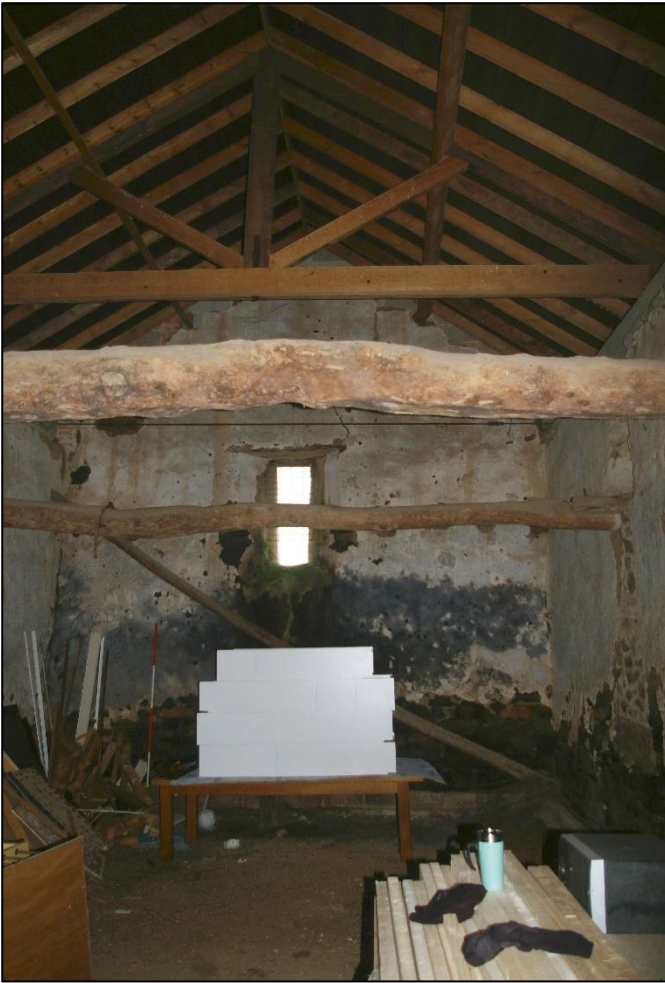
12. WESTERN PART OF CIDER BARN FROM EAST, WITH C18 LOFT FLOOR BEAMS AND C19 ROOF TRUSSES.
