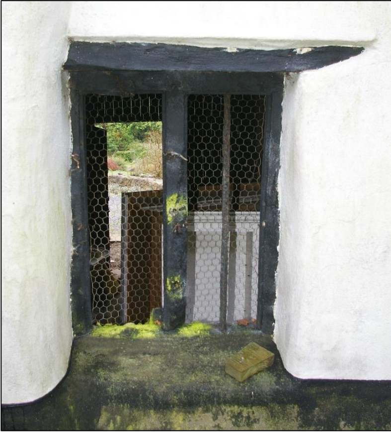
7. C18 WINDOW RE-USED IN C19 IN REAR WALL OF BARN, VIEW FROM NORTH.
