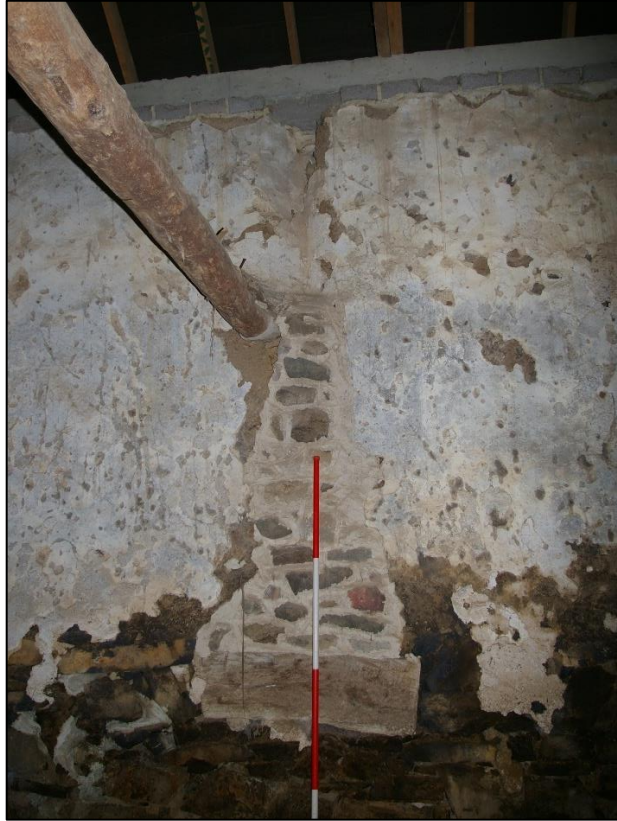
18. SITE OF WESTERN CRUCK FOOT IN NORTH WALL, WITH LARGE ELM PAD UNDER C19 RUBBLE PATCH. VIEW FROM SOUTH.
