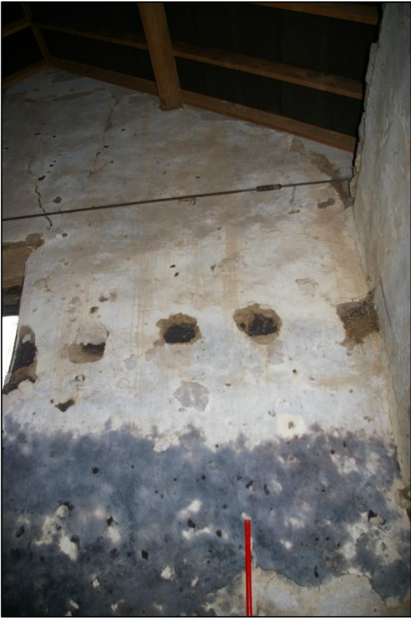
16. NORTH HALF OF WEST GABLE, LOOKING UP FROM EAST. NOTE OLD JOIST HOLES AND BLACK URINE-STAINING.
