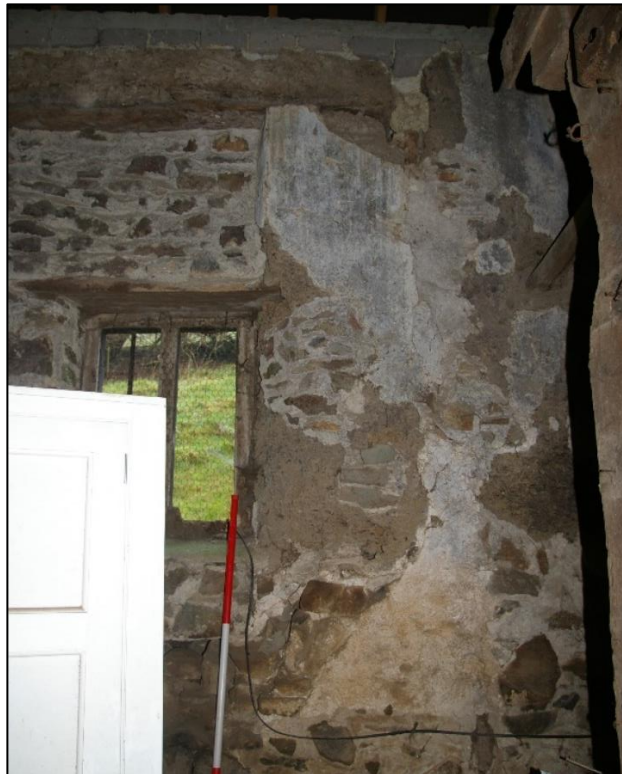
21. EAST JAMB OF NORTH THRESHING DOOR WITH EXTENSIVE C19 RUBBLE REPAIRS. VIEW FROM SOUTH.
