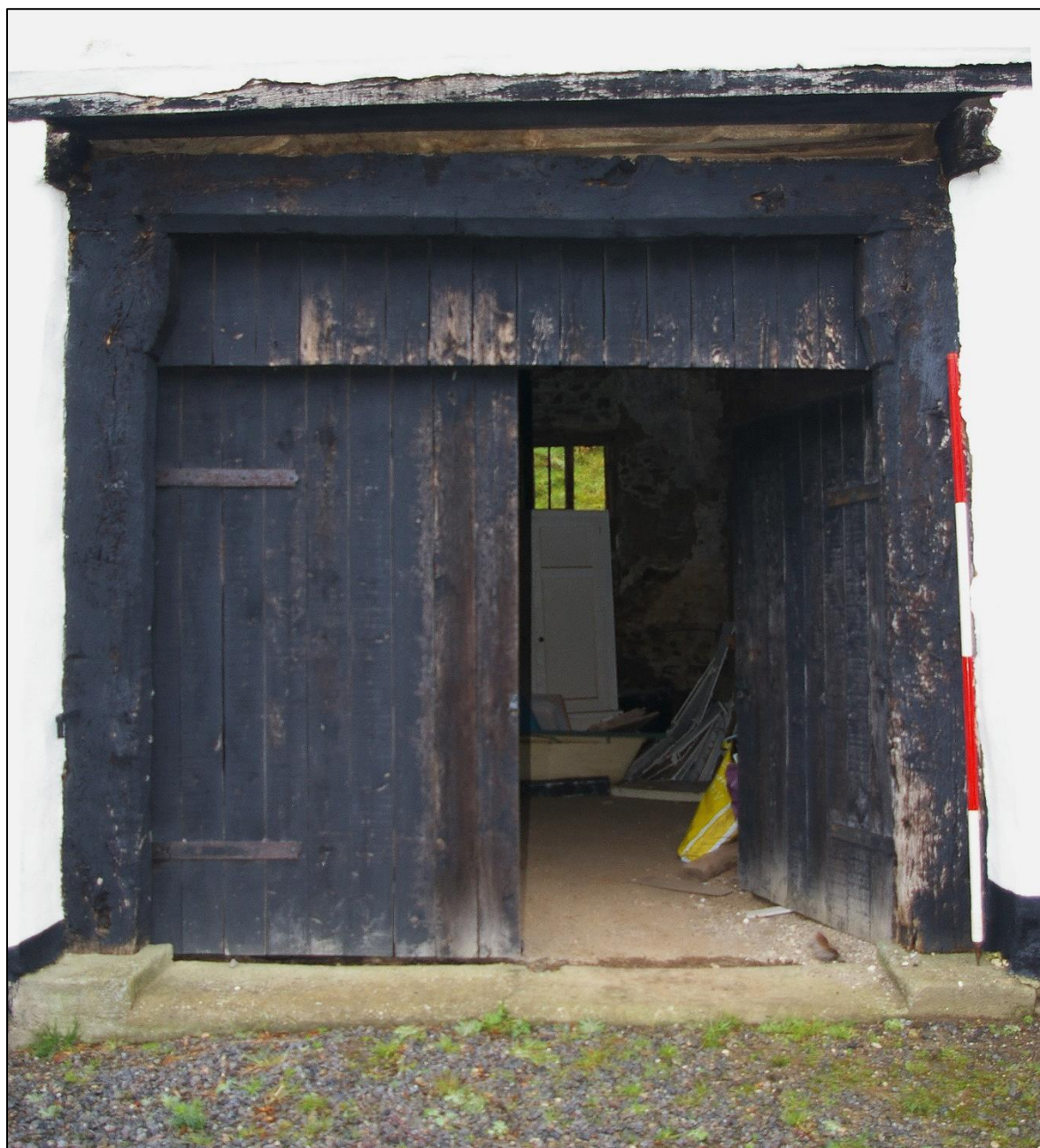
FIGURE 10: LATE MEDIEVAL FRAME OF SOUTHERN THRESHING DOOR WITH SHOULDERED POSTS; VIEW FROM SOUTH (2M SCALE).
