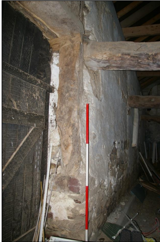
30. WEST JAMB OF THRESHING DOOR IN SOUTH WALL, WITH OAK CHEEK FORMERLY SUPPORTING DOOR LINTEL, FACE-PEGGED TO EAST FACE OF CRUCK FOOT. NOTE BARK AT BOTTOM RIGHT OF CHEEK.
