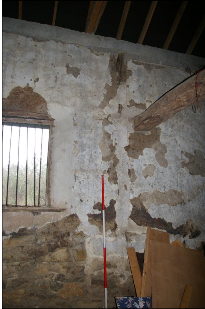
34. WESTERN CRUCK FOOT IN SOUTH WALL, VISIBLE AS VERTICAL MARK IN PLASTER. VIEW FROM NORTH.
