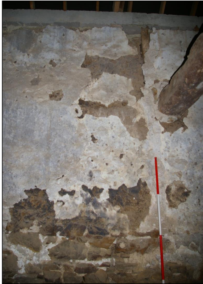
32. SOUTH WALL AT SECOND CRUCK TRUSS FOOT FROM WEST. VIEW FROM NORTH.
