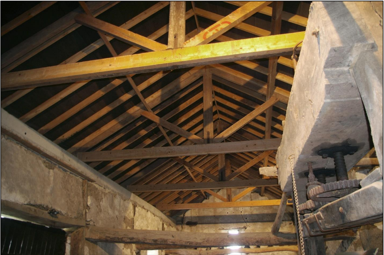
36. C19 ROOF STRUCTURE, REPAIRED AND REST ON CONCRETE EAVES COURSE IN LATE C20. LOOKING UP FROM EAST WITH C19 CIDER PRESS ON RIGHT.
