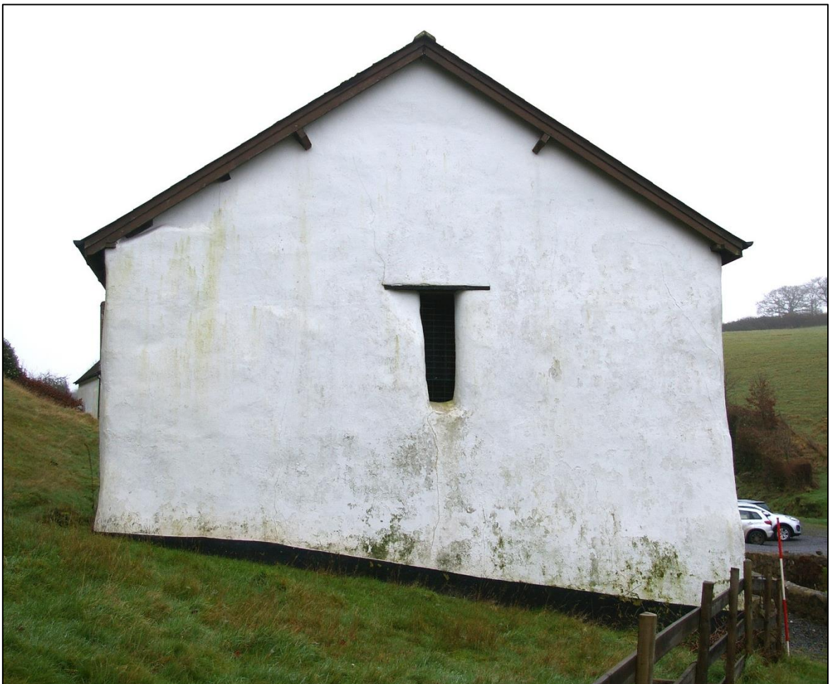
FIGURE 9: WEST END ELEVATION OF THE CIDER BARN SHOWING GROUND SLOPE; VIEW FROM WEST (2M SCALE).
