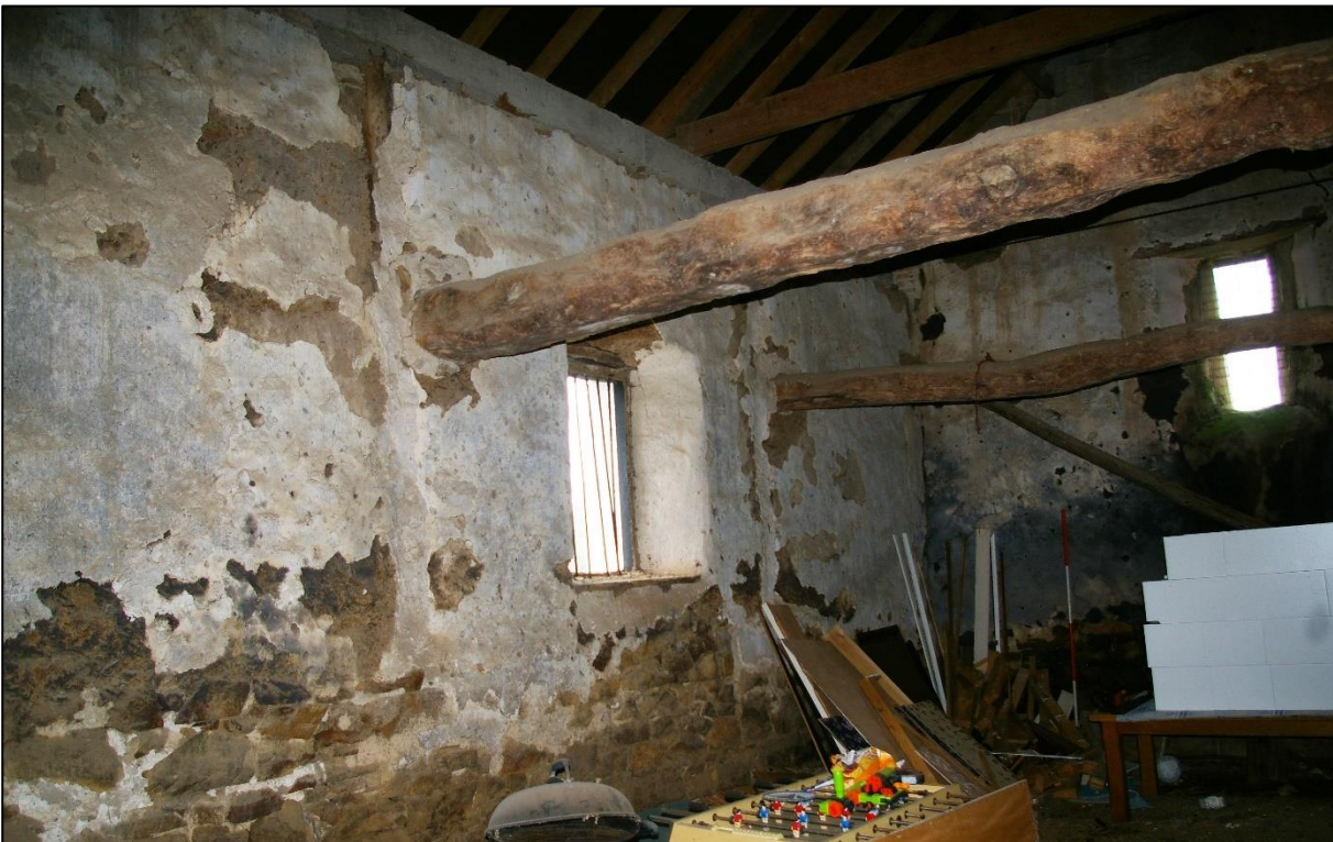
13. SOUTH WALL OF CIDER BARN TO WEST OF THRESHING DOOR, VIEWED FROM NORTH-EAST. VERTICAL INDENTATIONS SHOW POSITIONS OF CRUCK FEET, WITH C18 LOFT FLOOR BEAMS CUT INTO OLDER PLASTER.
