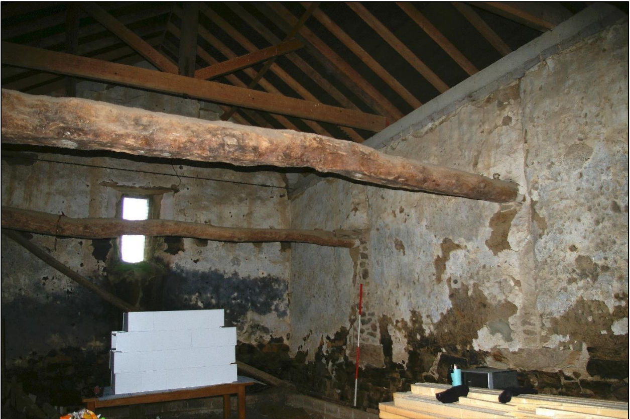
14. WEST END OF CIDER BARN FROM SOUTH-EAST, WITH GABLE WALL TO LEFT AND FIRST THREE BAYS OF NORTH WALL TO RIGHT.
