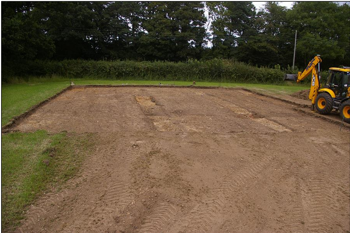
2. SITE SHOT, MID-EXCAVATION SHOWING INITIAL TRENCHES THROUGH STONY LAYERS; VIEWED FROM THE SOUTH (NO SCALE).
