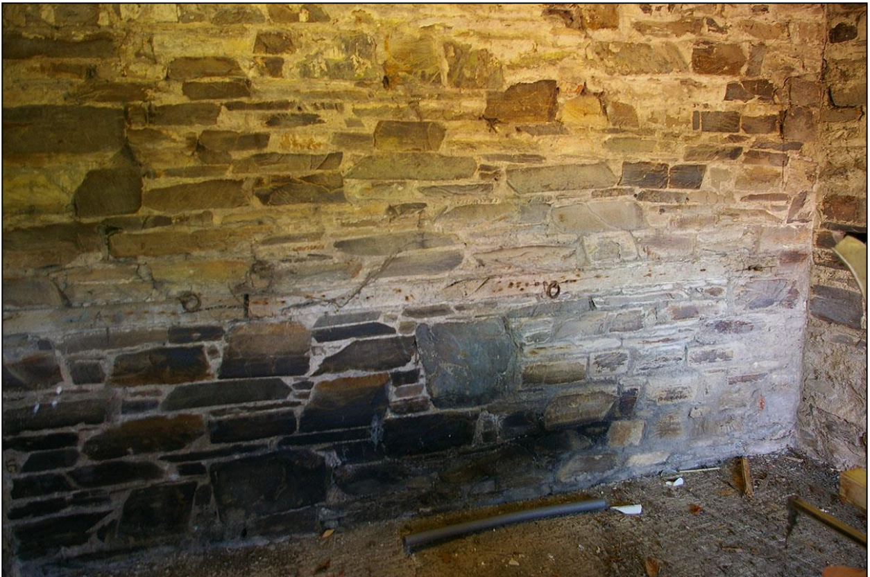
43. THE LONG TIMBER TIE SET LOW INTO THE SOUTH WALL, WITH ROW OF THREE RINGS; FROM THE NORTH-EAST.
