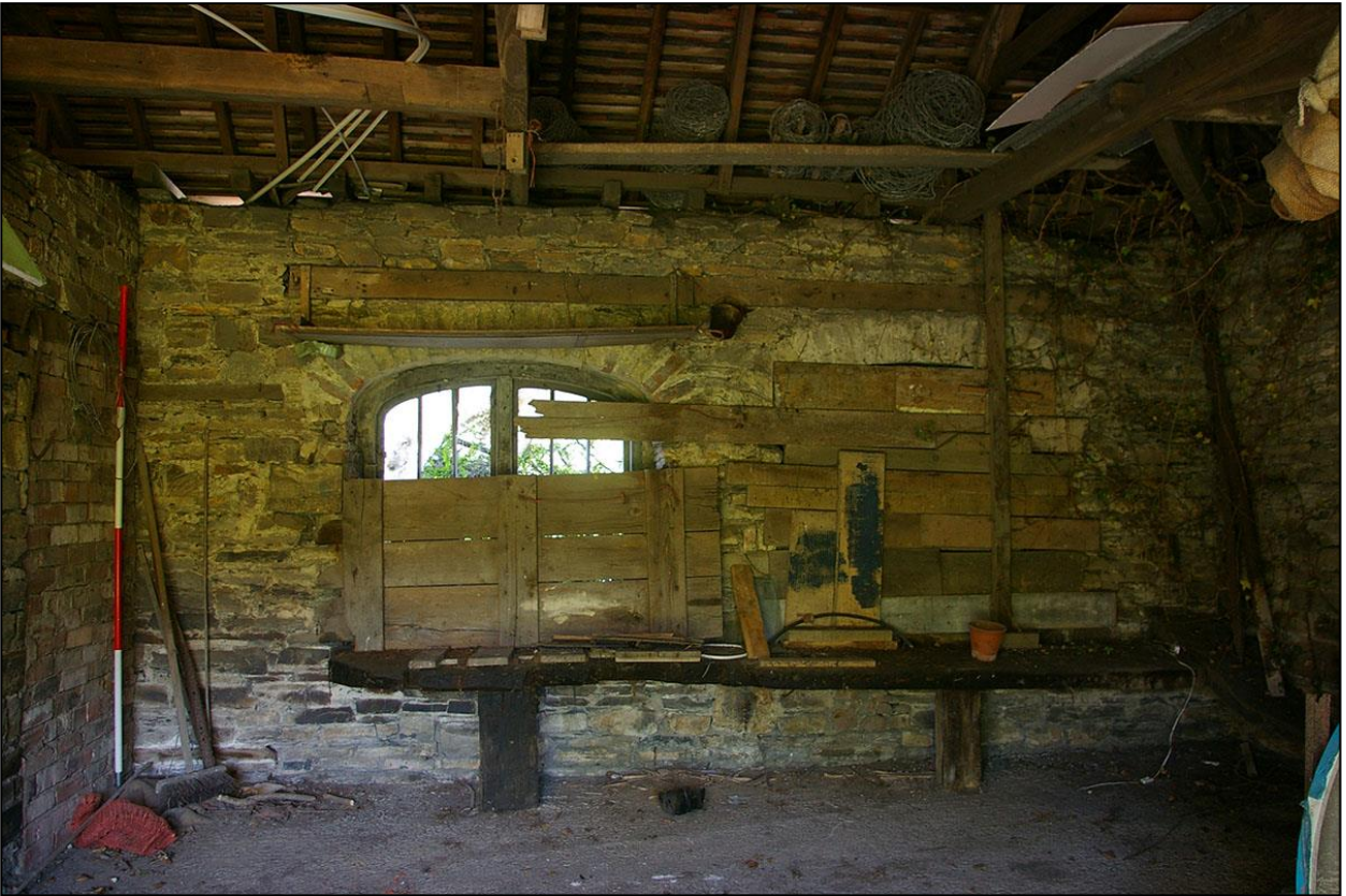
24. THE NORTH WALL OF ROOM 1, WITH 2M SCALE, WITH WINDOWS W1 & W2; FROM THE SOUTH.
