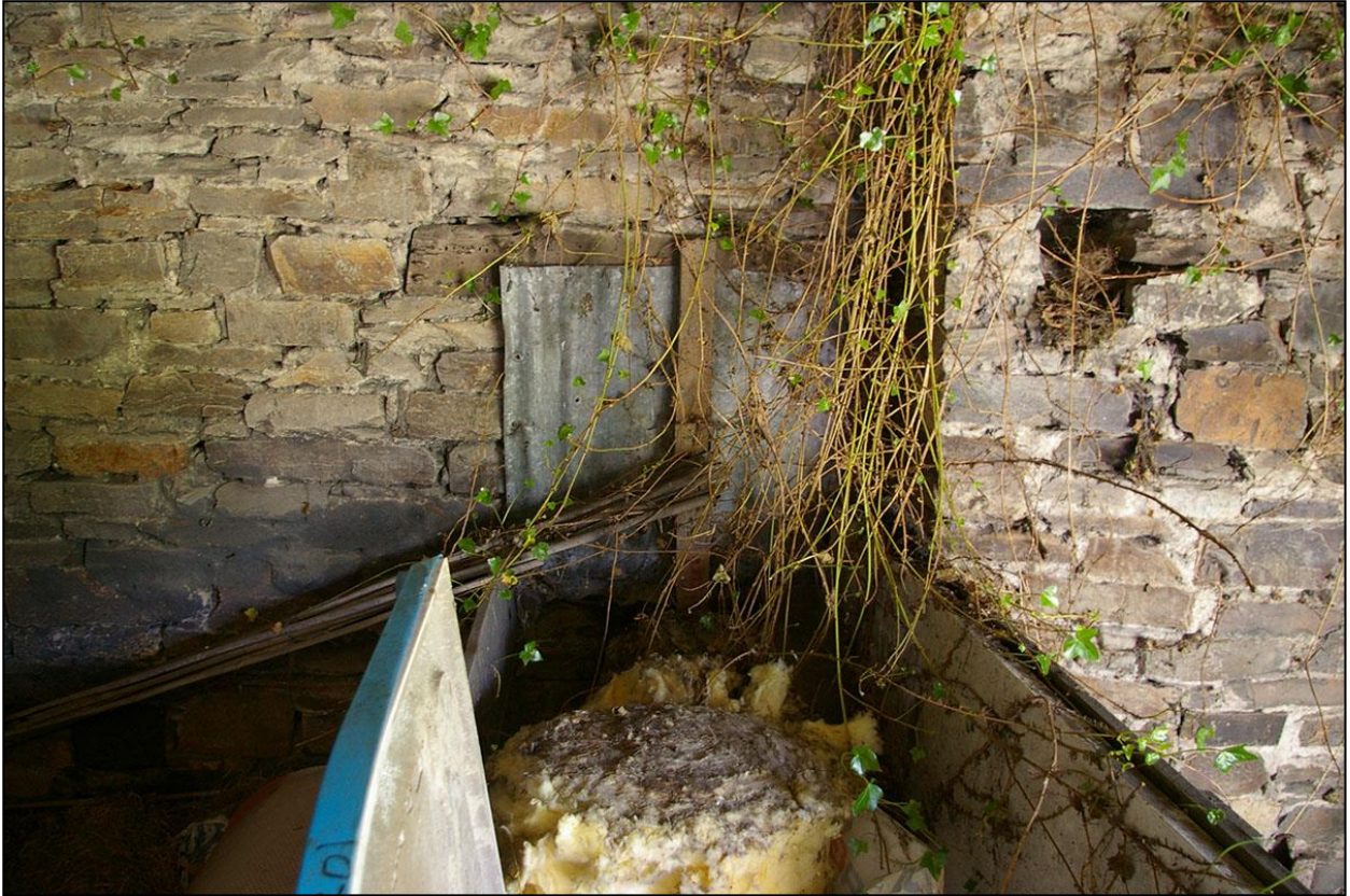
30. BD3 – THE BLOCKED OPENING IN THE EAST WALL, COVERED BY CORRUGATED SHEETING. DIRECTLY OPPOSITE BD2; FROM THE WEST.
