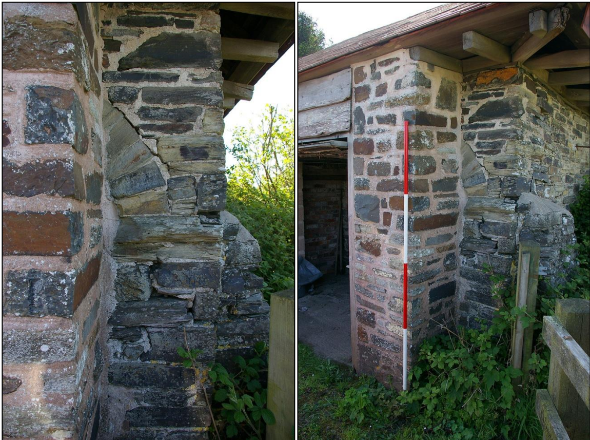
6. LEFT: THE SMALL SECTION OF THE SECOND ARCH TO THE NORTH ELEVATION, NORTH-WEST CORNER; FROM THE NORTH.
