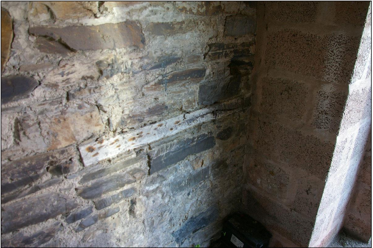
40. THE TIMBER TIE WITHIN THE WEST WALL, TO THE NORTH-WEST CORNER; FROM THE SOUTH-EAST.
