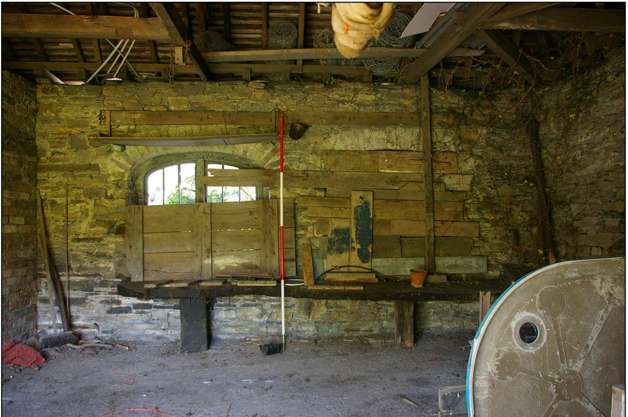
27. THE NORTH WALL OF ROOM 1, SHOWING WORKBENCH, WITH 2M SCALE; FROM THE SOUTH.
