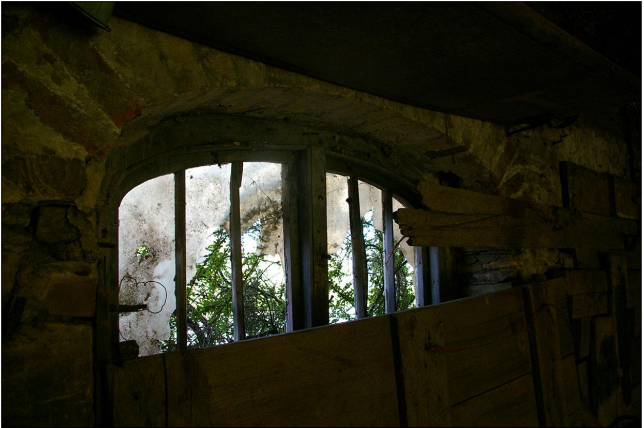
26. W2, SHOWING THE DETAIL OF THE WINDOW FRAME WITHIN THE OPENING; FROM THE SOUTH-WEST.
