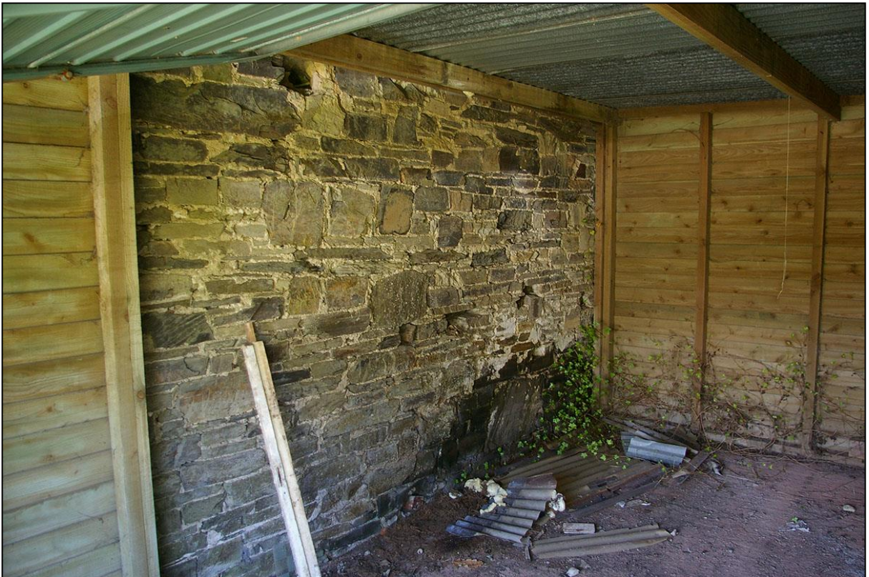
35. THE REAR WALL OF THE SMITHY, FROM WITHIN THE GARAGE, ROOM 3; FROM THE SOUTH-WEST.
