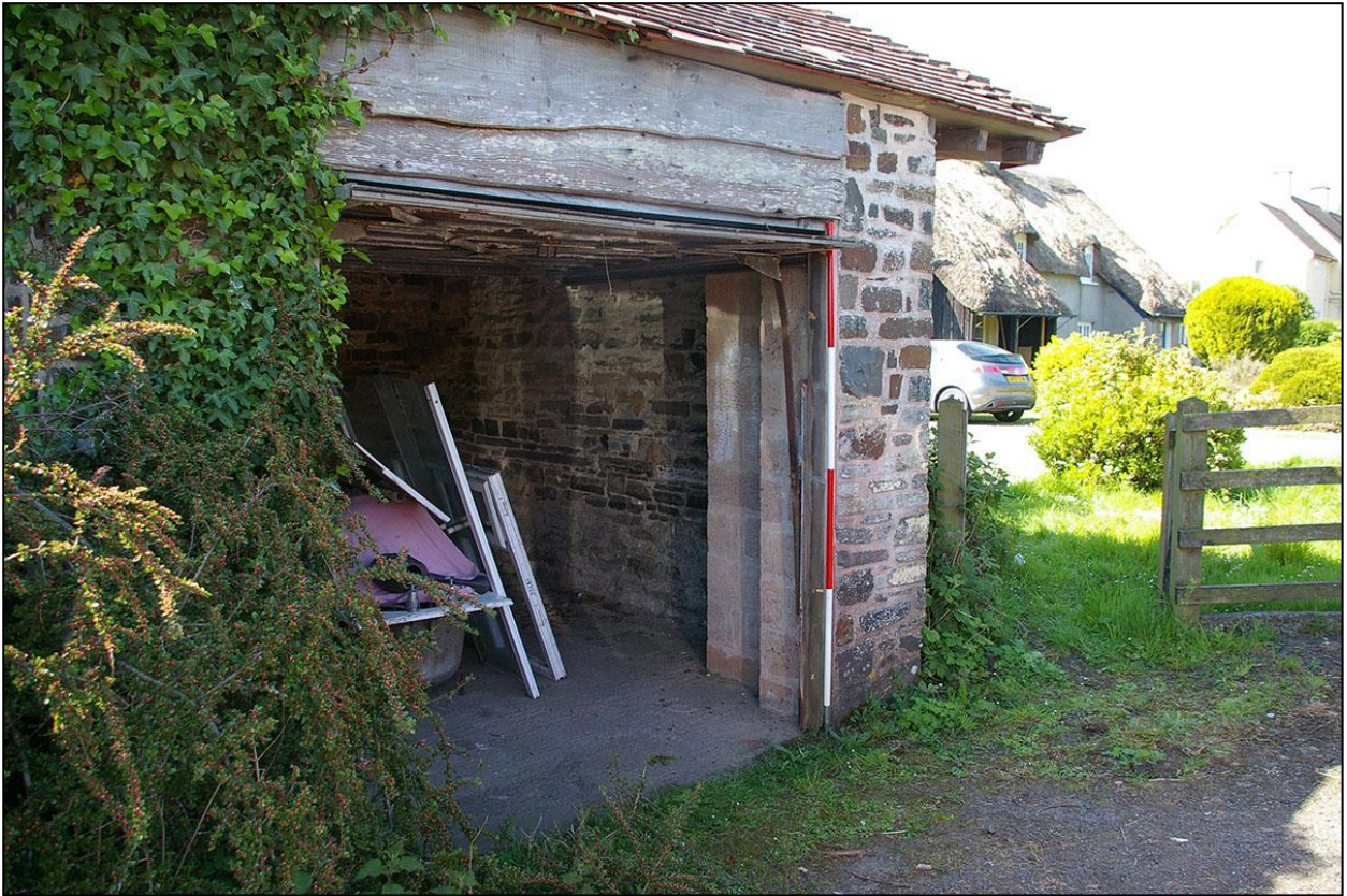
5. THE LARGE GARAGE OPENING, D2, FORCED INTO THE FRONT NORTH ELEVATION, WITH 2M SCALE; FROM THE NORTH-EAST.
