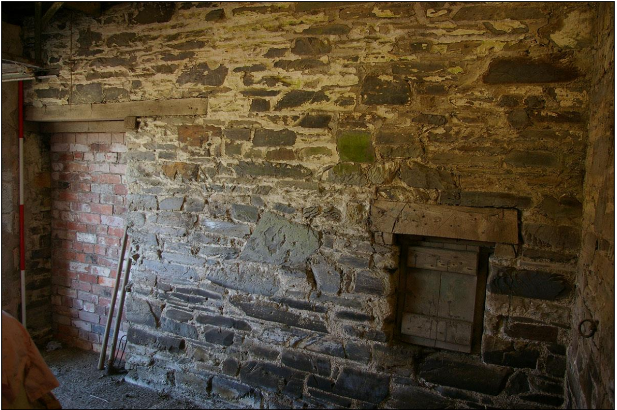
44. THE PARTY WALL TO THE EAST OF ROOM 1, WITH 2M SCALE, WITH OPENINGS; FROM THE SOUTH-WEST.
