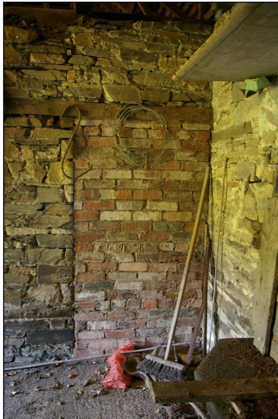
23. BD1 – THE BLOCKED DOORWAY IN THE WEST WALL OF ROOM 1; FROM THE EAST.
