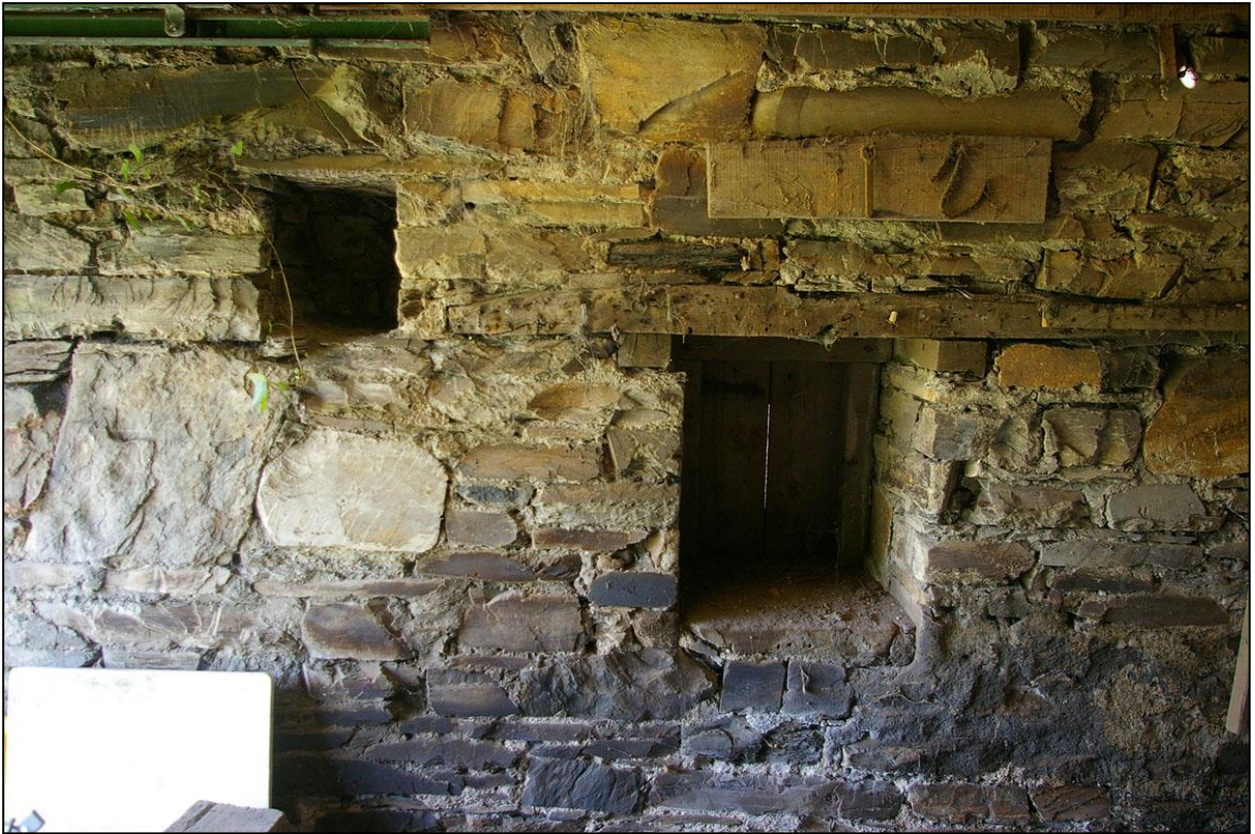
20. THE TWO OPENINGS IN THE WEST WALL OF ROOM 1; FROM THE EAST.
