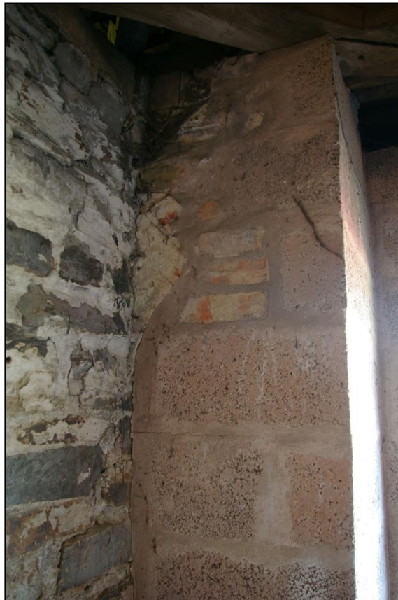
39. THE INNER PART OF THE ARCH ON THE NORTH-WEST CORNER; FROM THE SOUTH-EAST.
