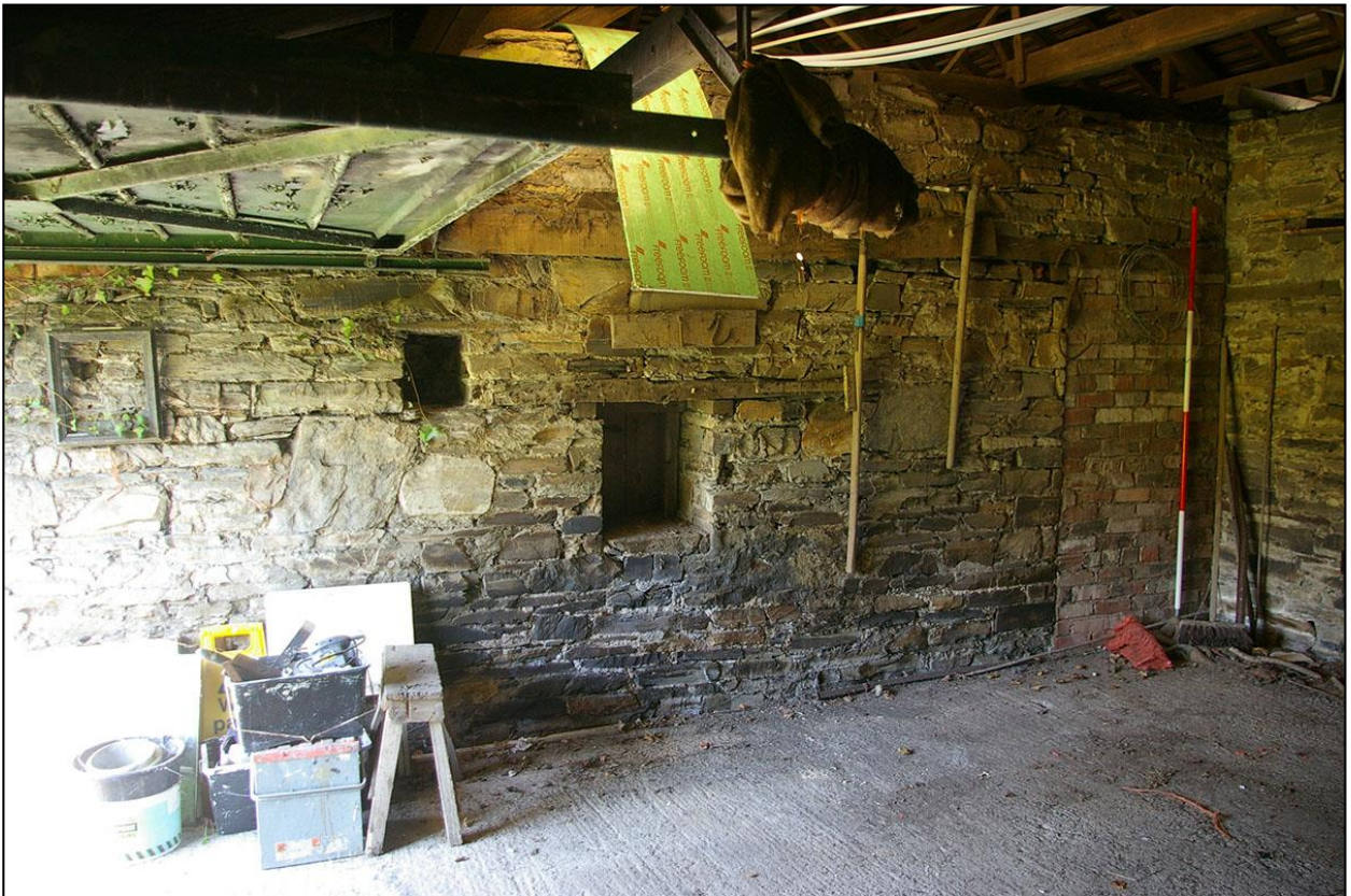
19. THE WEST PARTY WALL, FROM WITHIN ROOM 1, WITH 2M SCALE; FROM THE SOUTH-EAST.
