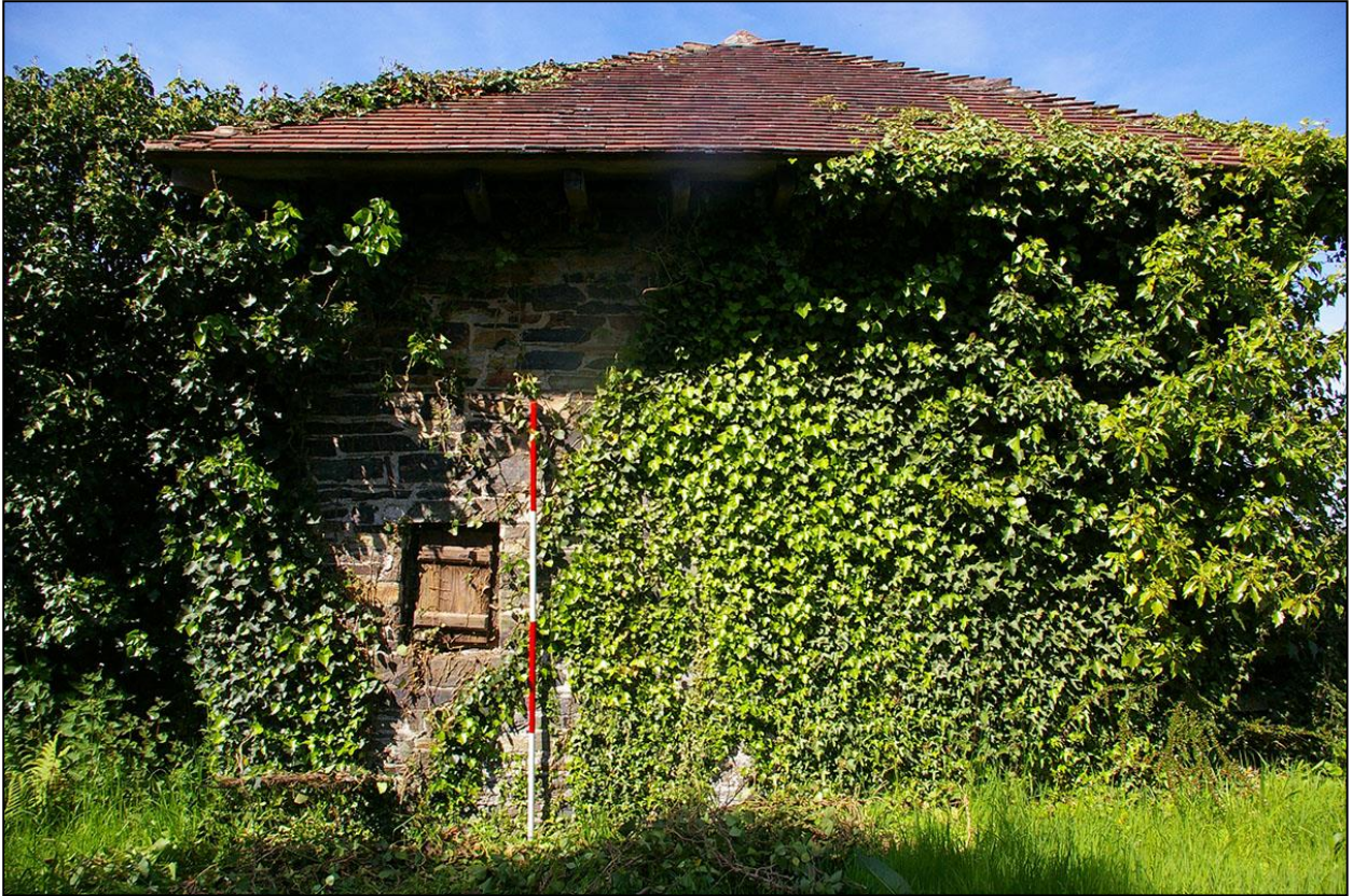
16. THE EAST ELEVATION OF THE SMITHY, WITH 2M SCALE; FROM THE EAST.
