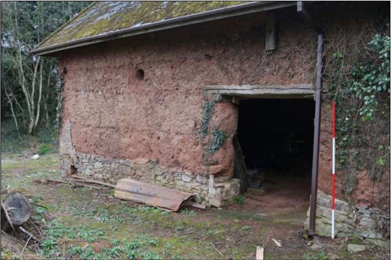
3. THE NORTH WALL OF B1, SHOWING THE RAISES IN THE COB; VIEWED FORM THE NORTH-WEST (SCALE 9M).
