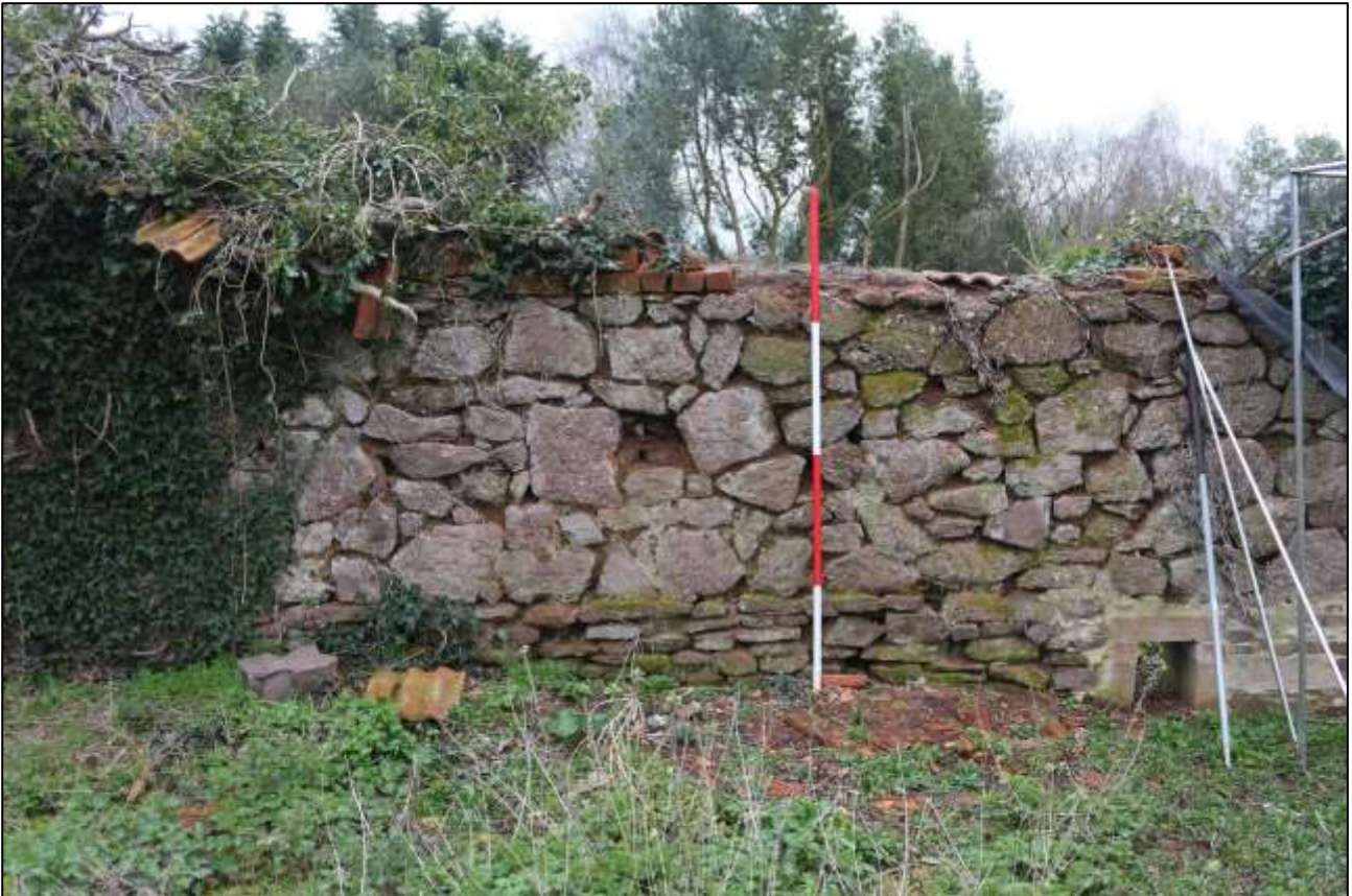
11. DETAIL OF THE REAR (WEST) WALL OF B2, SHOWING THE DIFFERENT STONE USED FOR THE RAISE; VIEWED FROM THE WEST (SCALE 2M).
