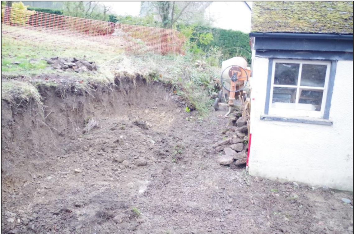
3. WORKING SHOT, OF WORKS AS THEY PROGRESSED, VIEWED FROM THE EAST (1M SCALE).
