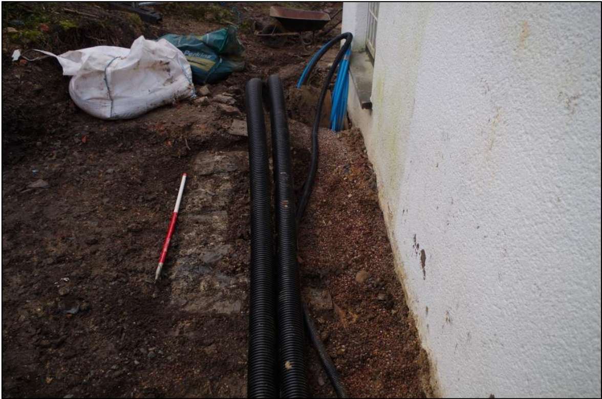
FIGURE 7: FOOTING OF STRUCTURE TO EAST OF BIDGOODS, VIEWED FROM THE NORTH (1M SCALE).
