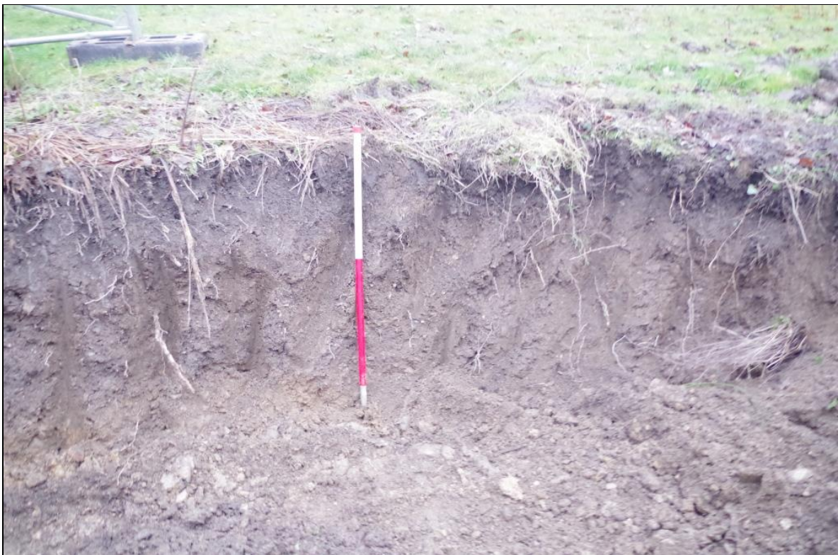
2. EDGE OF EXCAVATION TO THE SOUTH OF THE EXTENSION, VIEWED FROM THE SOUTH (1M SCALE).
