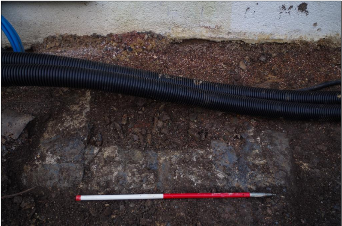
11. FOOTING OF STRUCTURE TO EAST OF BIDGOODS, VIEWED FROM THE EAST (1M SCALE).
