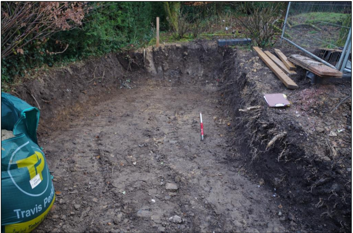
10. LIMITS OF EXCAVATION TO THE EAST OF BIDGOODS, VIEWED FROM THE WEST (1M SCALE).
