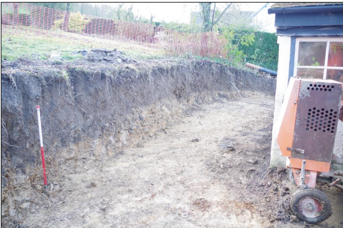
4. AS ABOVE AT COMPLETION OF EXCAVATIONS, VIEWED FROM THE EAST (1M SCALE).
