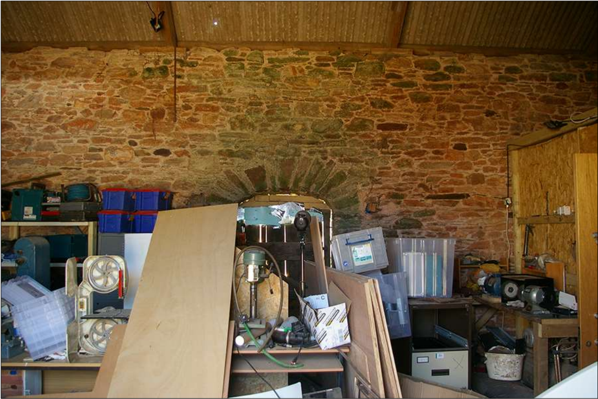
98. THE INTERIOR FACE OF THE SOUTH-WEST WALL OF B2 SHOWING THE FINE SEGMENTAL ARCH, VOISSIORS AND KEYSTONE OVER LOADING DOOR D9; VIEWED FROM THE NORTH-EAST.
