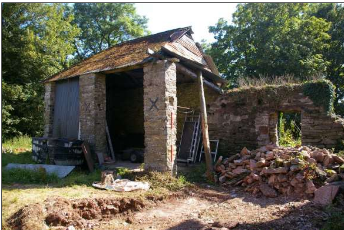
FIGURE 10: LINHAY B3, DEMONSTRATING THE COLLAPSED NORTH-WESTERN END; VIEWED FROM THE NORTH (2M SCALE).
