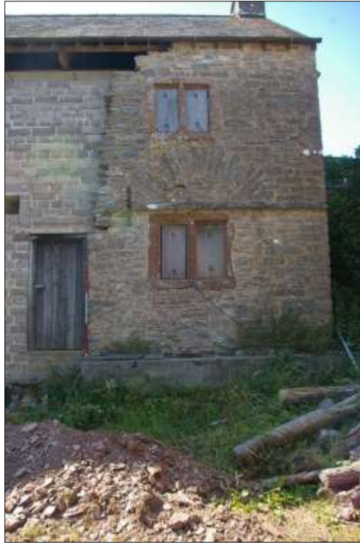
25. DETAIL OF THE SOUTH-EAST ELEVATION OF B1, SHOWING THE SURVIVING HISTORIC FABRIC; VIEWED FROM THE SOUTH-EAST (2M SCALE).
