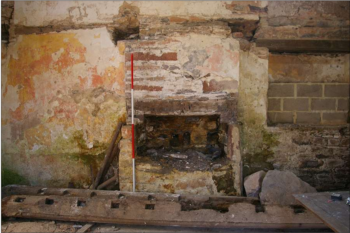
46. DETAIL OF FIREPLACE FP1 IN THE NORTH-WEST WALL OF THE SOUTH-WEST GROUND-FLOOR ROOM OF B1; VIEWED FROM THE SOUTH-EAST (2M SCALE).
