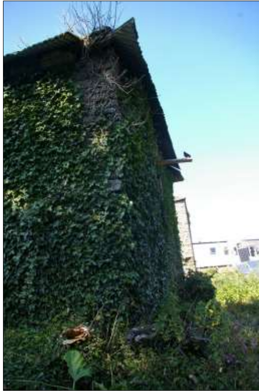
107. DETAIL OF THE SOUTH-EASTERN CORNER OF THE SOUTH-WEST AND SOUTH-EAST ELEVATIONS OF B3; VIEWED FROM THE SOUTH-SOUTH-WEST.
