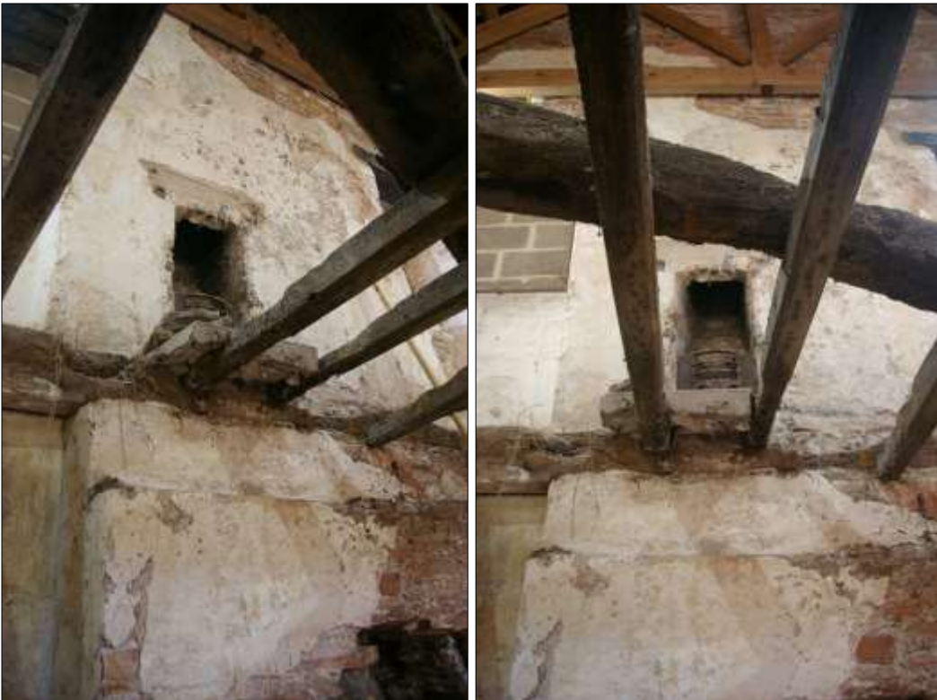
84. (LEFT) DETAIL OF FIREPLACE FP3 IN THE NORTH-EAST WALL OF THE NORTH-EAST FIRST-FLOOR ROOM WITHIN B1; VIEWED FROM THE WEST.
