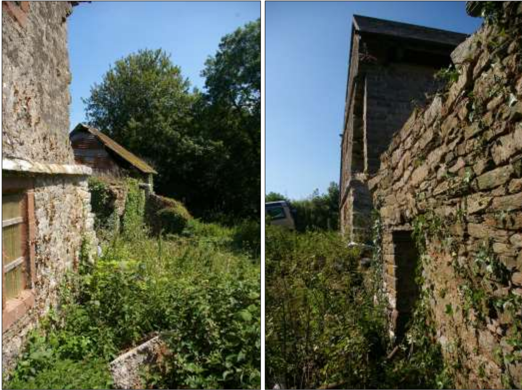
22. (LEFT) VIEW ALONG THE FULL SOUTH-WEST ELEVATION OF B1 AND B3 DEMONSTRATING THE PARTIALLY COLLAPSED BUT COHESIVE NATURE OF THE WALLS; VIEWED FROM THE WEST.
