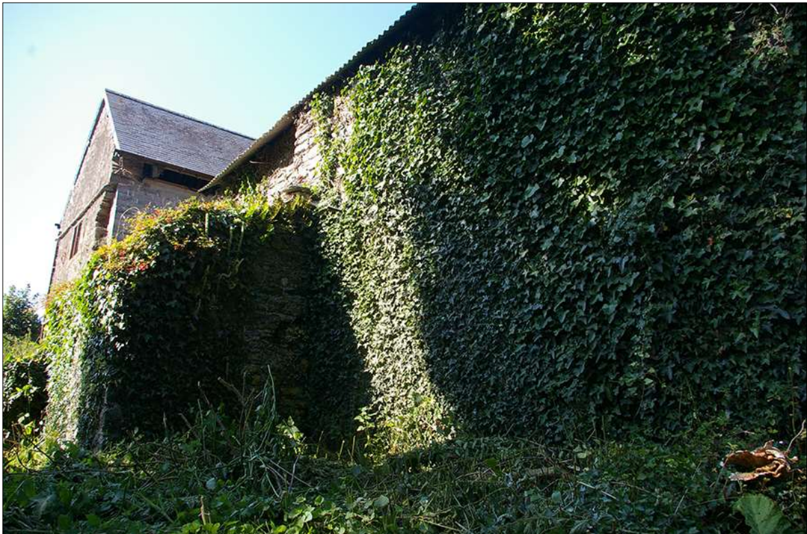
106. THE SOUTH-EASTERN END OF THE SOUTH-WEST ELEVATION OF B3; VIEWED FROM THE SOUTH-SOUTH-EAST.
