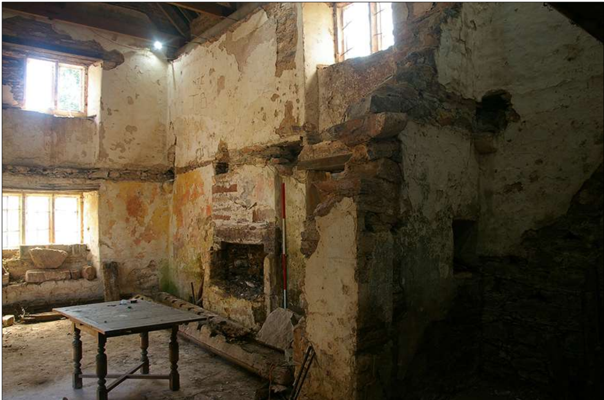
30. THE INTERIOR FACE OF THE NORTH-WEST WALL OF B1, SOUTH-WEST END; VIEWED FROM THE EAST (2M SCALE).
