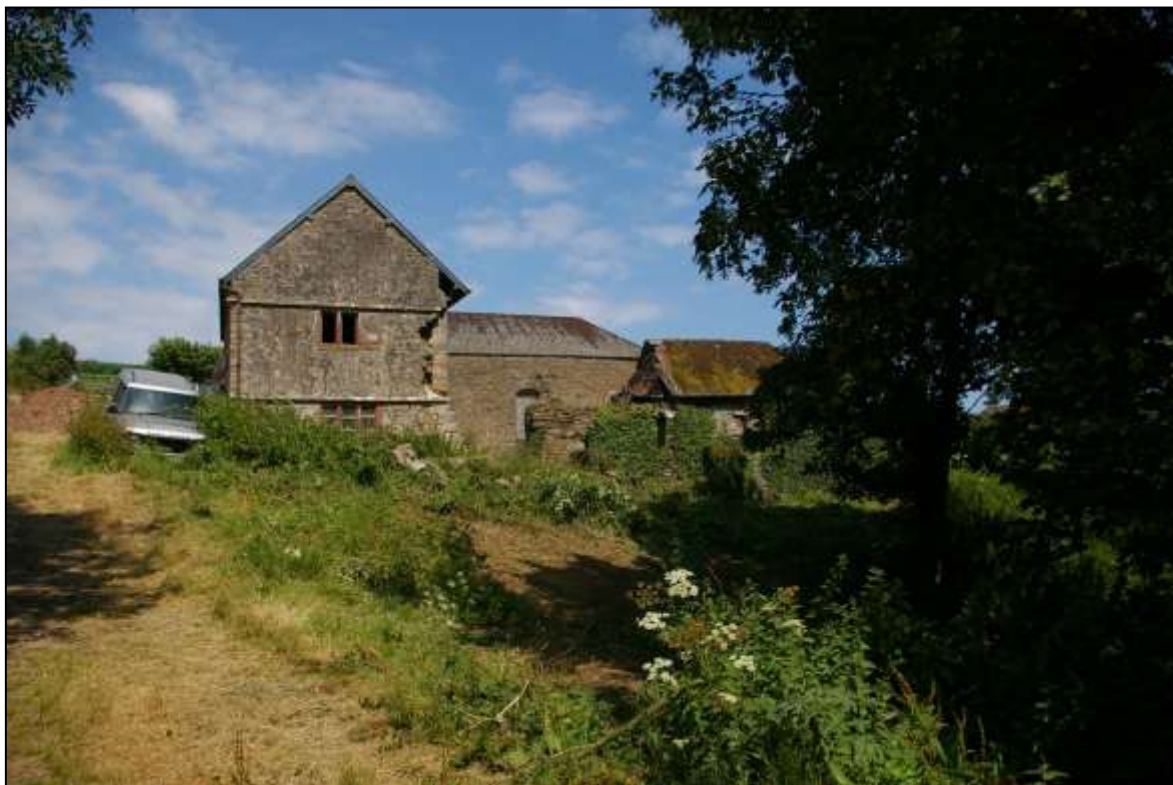
FIGURE 2: VIEW OF THE BUILDINGS AT WEEK, WITH B1 (LEFT), B2 (REAR CENTRE) AND B3 (RIGHT); VIEWED FROM THE SOUTH-WEST.
