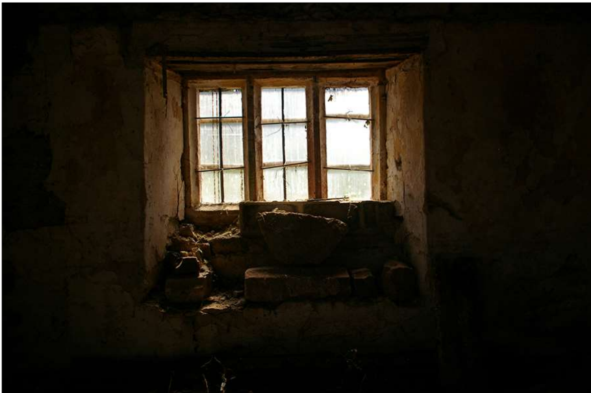
43. DETAIL OF THE INTERIOR FACE OF WINDOW W5 IN THE SOUTH-WEST WALL OF B1; VIEWED FROM THE NORTH-EAST.
