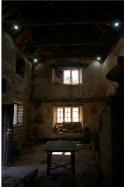
42. THE INTERIOR FACE OF THE SOUTH-WEST WALL WITH WINDOWS W5 AND W6; VIEWED FROM THE NORTH-WEST.
