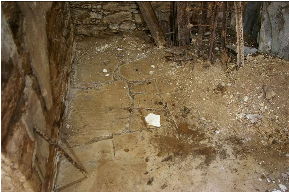
61. DETAIL OF SLATESTONE FLAG FLOOR BENEATH THE CONCRETE FLOOR OF THE NORTH-EAST GROUND-FLOOR ROOM OF B1; VIEWED FROM THE SOUTH-EAST.
