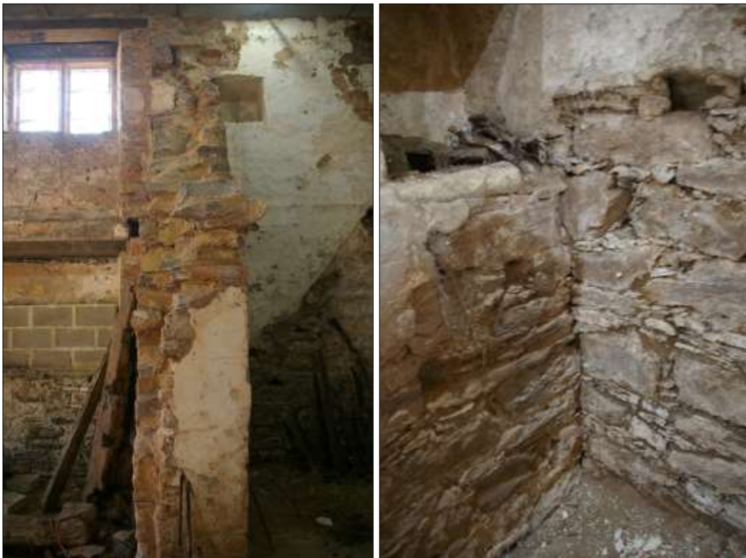
72. (LEFT) DETAIL OF THE PROFILE OF THE SURVIVING SECTION OF CROSS-WALL BETWEEN THE TWO GROUND-FLOOR ROOMS OF B1, NOTE THE PLASTER INDICATING THE PRESENCE OF A DOORWAY AT THIS POINT; VIEWED FROM THE SOUTH-EAST.
