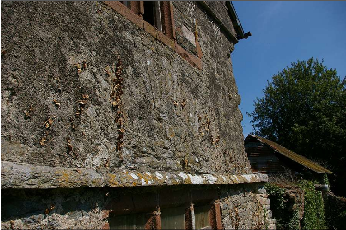
20. DETAIL OF THE SLATESTONE SLAB SEGMENTAL POINTED ARCH OVER W5 IN THE SOUTH-WEST ELEVATION OF B1; VIEWED FROM THE WEST.
