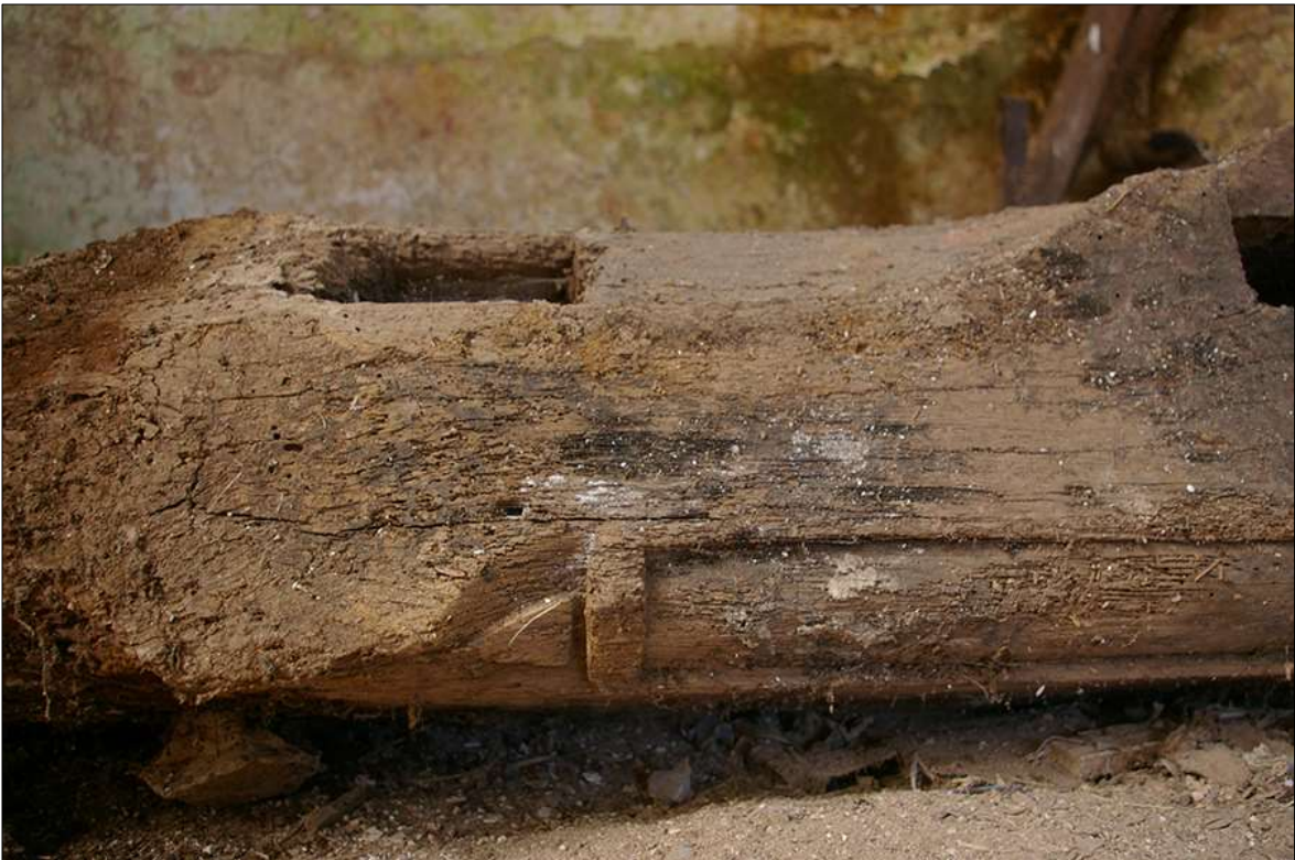
55. DETAIL OF THE BAR AND CUT STOP ON THE EX SITU FINE OVOLO CARVED BEAM; VIEWED FROM THE SOUTH-EAST.
