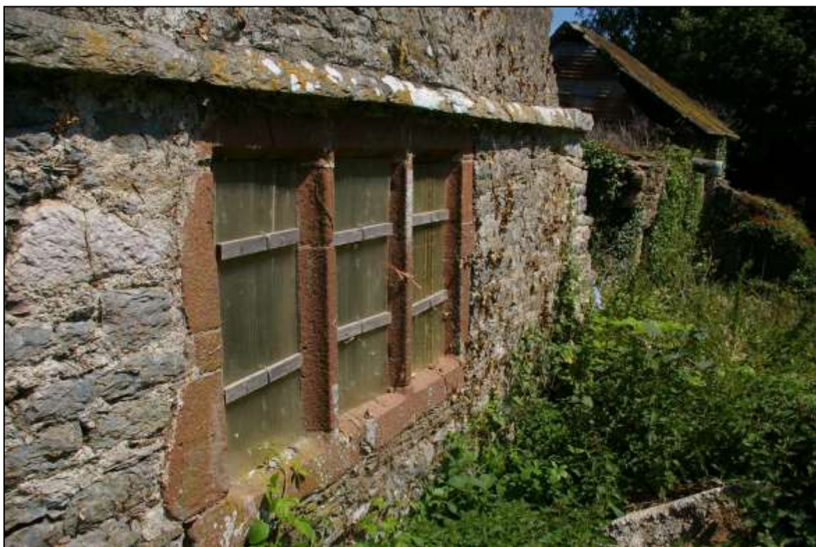
FIGURE 5: EXAMPLE OF THE RE-USED RED SANDSTONE WINDOW MULLIONS, IN THIS CASE FOR WINDOW W5 IN THE SOUTH-WEST ELEVATION OF B1; VIEWED FROM THE WEST.
