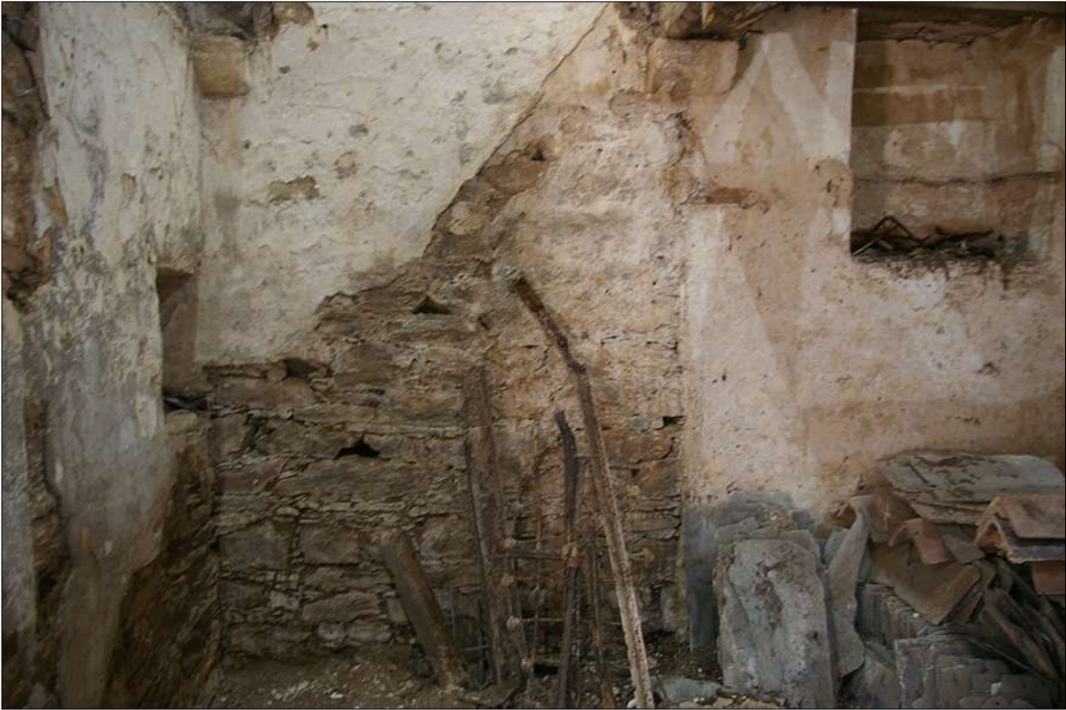
76. DETAIL OF THE SCAR OF THE FORMER STAIR AGAINST THE NORTH-WEST WALL OF THE NORTH-EAST GROUND-FLOOR ROOM WITHIN B1; VIEWED FROM THE SOUTH-EAST.
