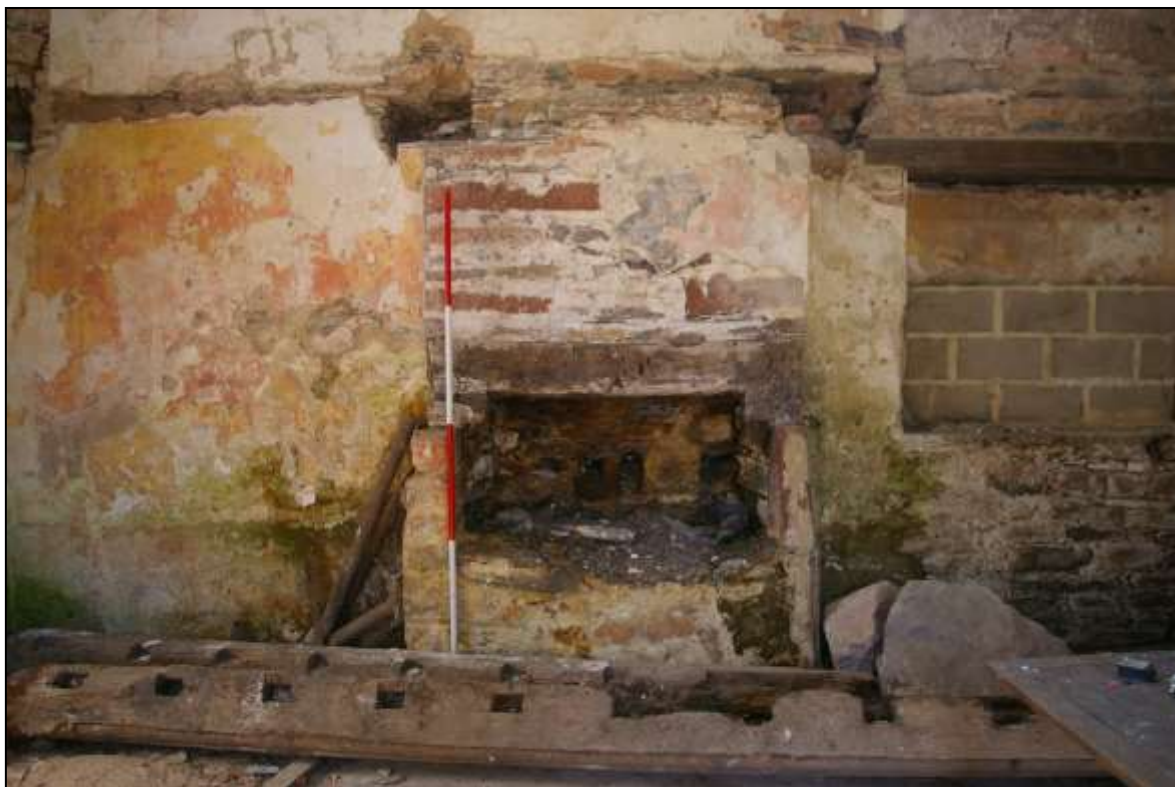
FIGURE 7: DETAIL OF FIREPLACE FP1 WITHIN THE SOUTH-WESTERN GROUND-FLOOR ROOM OF B1; VIEWED FROM THE SOUTH-EAST (2M SCALE).
