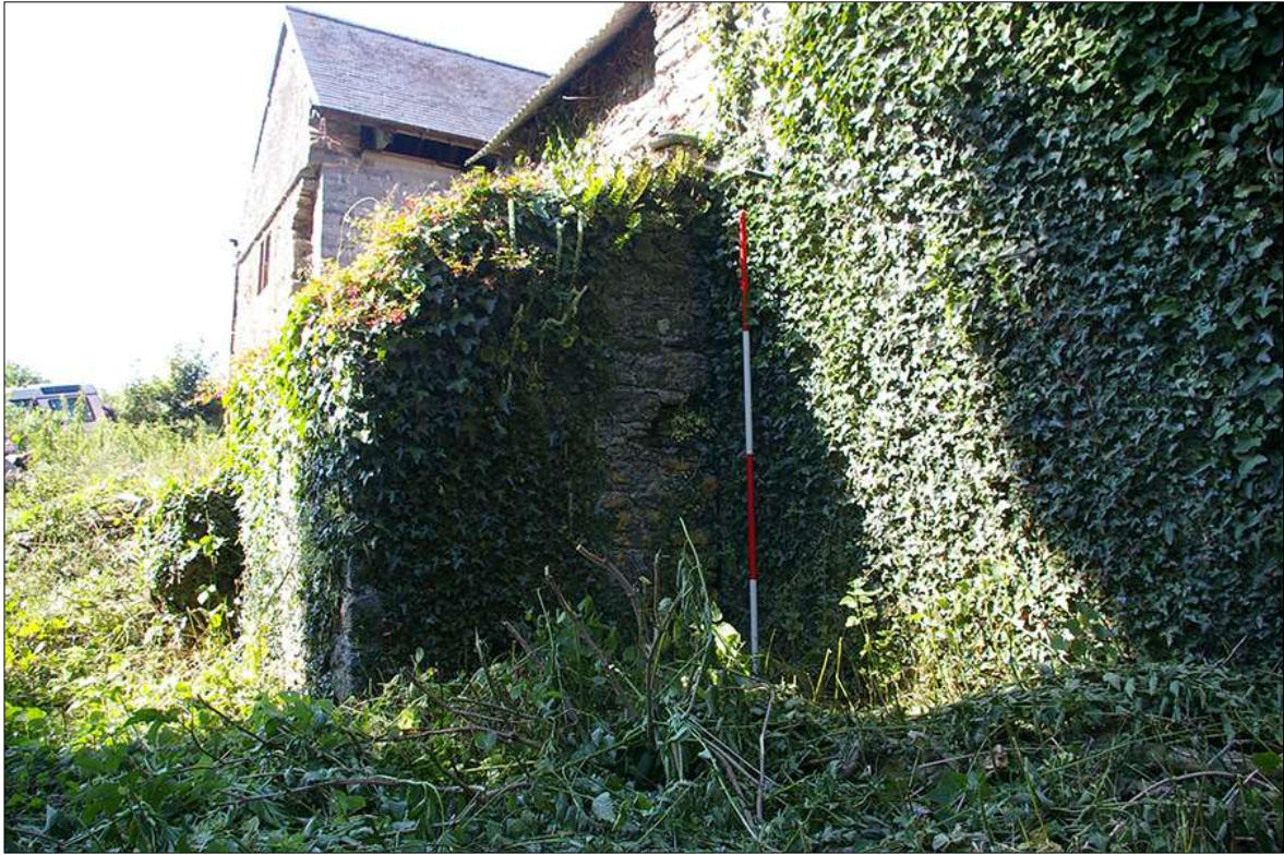
105. THE SOUTH-EAST AND SOUTH-WEST ELEVATIONS OF THE POSSIBLE 'GARDEROBE'; VIEWED FROM THE SOUTH-SOUTH-EAST (2M SCALE).
