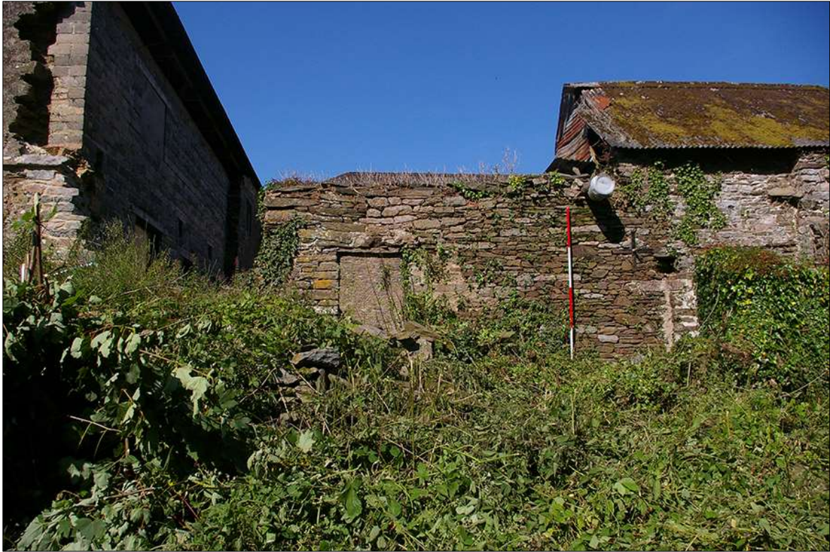
102. DETAIL OF THE DIFFERING BUILDS WITHIN THE SOUTH-WEST ELEVATION OF B3; VIEWED FROM THE SOUTH-WEST (2M SCALE).
