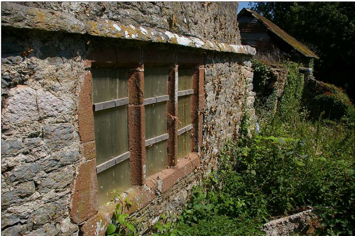
19. DETAIL OF WINDOW W5 IN THE SOUTH-WEST ELEVATION OF B1; VIEWED FROM THE WEST.
