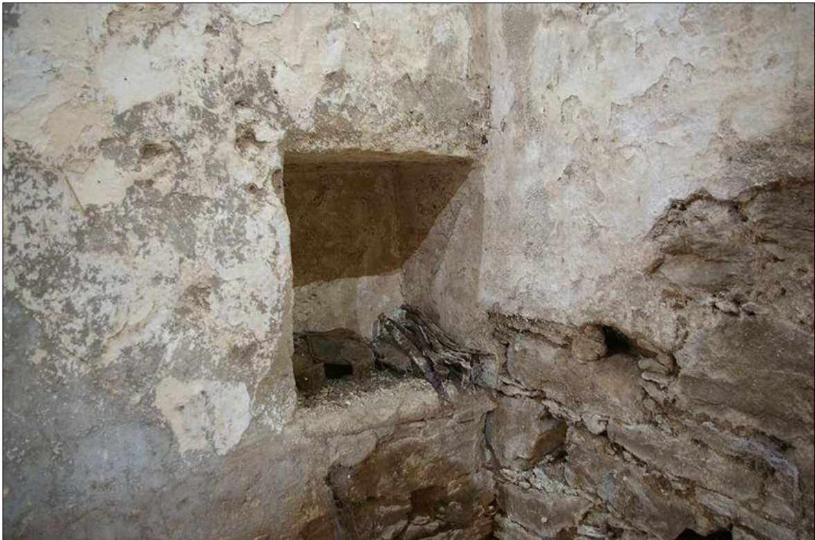
75. DETAIL OF THE SQUARE ALCOVE IN THE ANGLE OF THE CROSS-WALL AND NORTH-WEST WALL OF B1; VIEWED FROM THE EAST.
