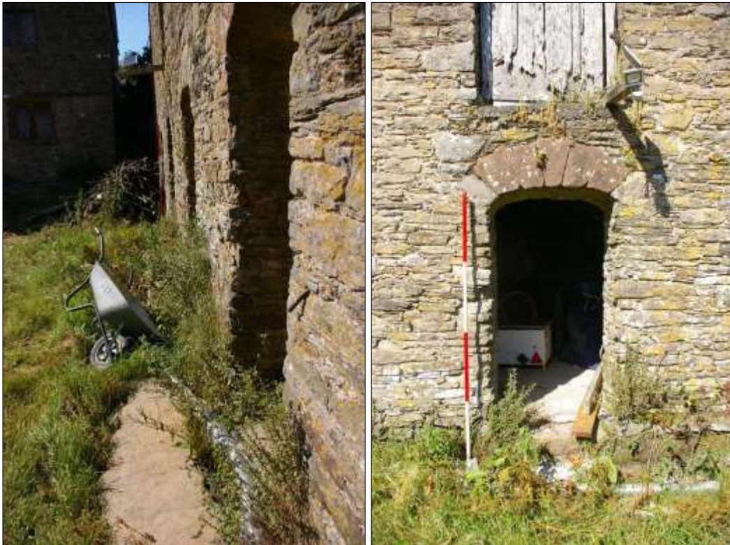
87. (LEFT) DETAIL OF THE SOUTH-WEST ELEVATION OF B2 DETAILING THE SLIGHTLY BATTERED ANGLE OF THE LOWER, HEAVIER STONEMWORK; VIEWED FROM THE SOUTH-SOUTH-EAST.
