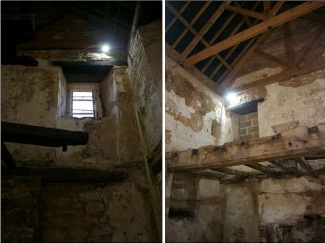
82. (LEFT) DETAIL WINDOW W1 WITH ITS RAILWAY SLEEPER LINTEL; VIEWED FROM THE SOUTH-WEST.
