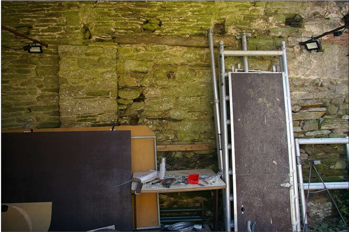
115. DETAIL OF BLOCKED DOORWAY D11 IN THE SOUTH-WEST ELEVATION OF B3; VIEWED FROM THE NORTH-EAST.
