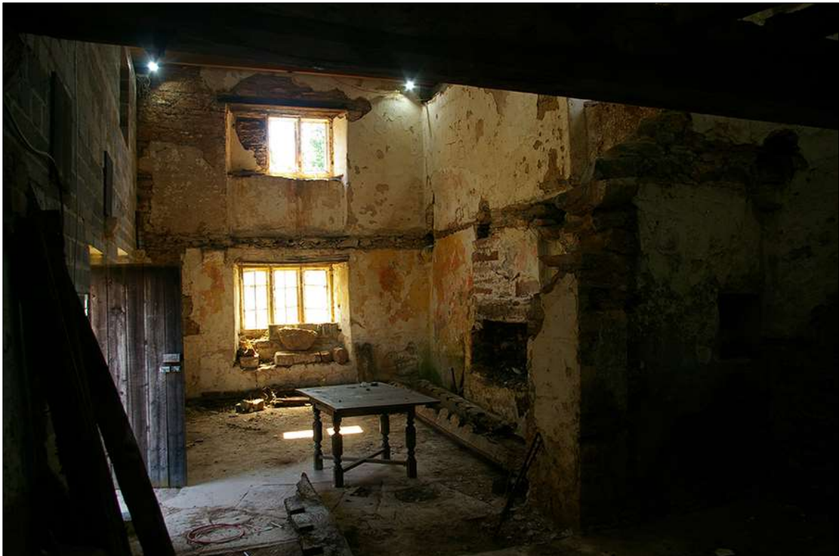
38. VIEW OF THE LARGER SOUTH-WESTERN GROUND-FLOOR ROOM WITHIN B1, DETAILING THE WINDOWS W5 AND W6, AND FIREPLACE FP1; VIEWED FROM THE NORTH-EAST.
