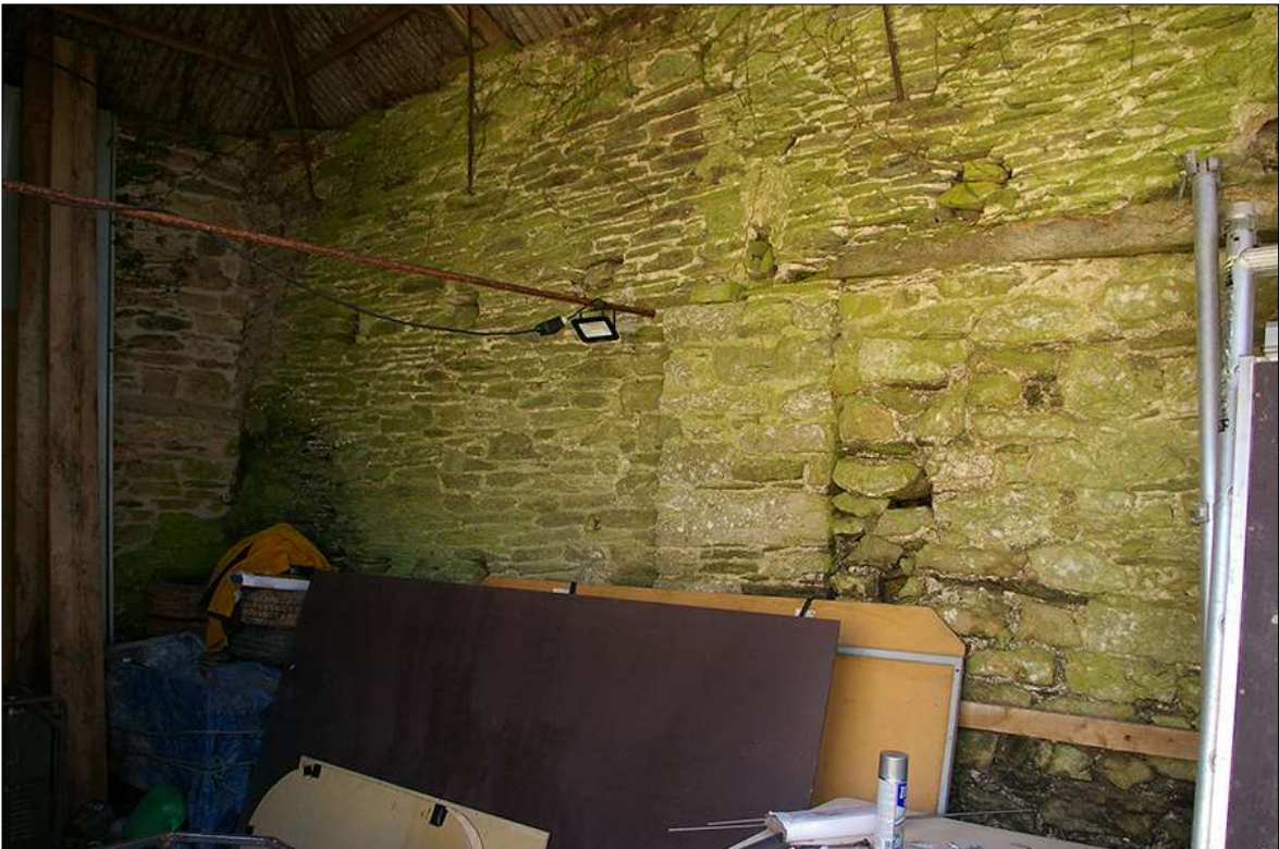
114. INTERIOR FACE OF THE SOUTH-WEST ELEVATION (SOUTH-EAST END) OF B3; VIEWED FROM THE NORTH.
