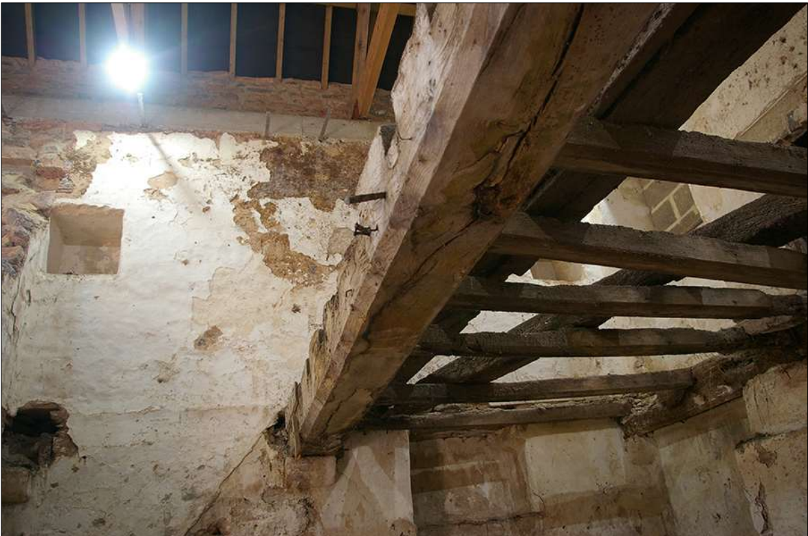
77. DETAIL OF THE SURVIVING CEILING BEAM TO THE NORTH-EAST GROUND FLOOR ROOM OF B1; VIEWED FROM THE EAST-SOUTH-EAST.
