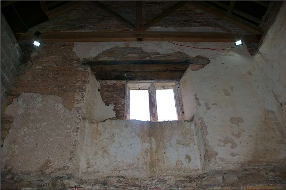
44. DETAIL OF THE INTERIOR FACE OF WINDOW W6 IN THE SOUTH-WEST WALL OF B1; VIEWED FROM THE NORTH-EAST.
