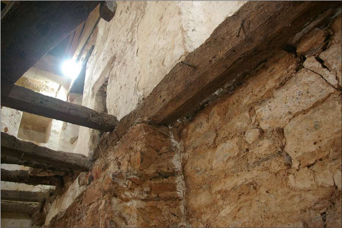
65. DETAIL OF FIREPLACE FP2, SHOWING THE CRUDE BUILD TO FIT IT AROUND THE CHAMFERED CEILING BEAM; VIEWED FROM THE SOUTH.
