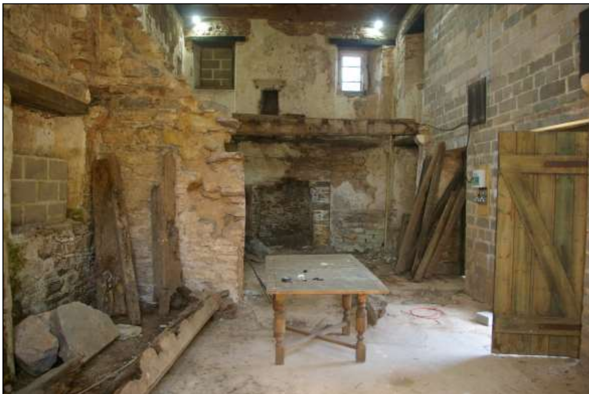
FIGURE 6: INTERIOR OF B1, SHOWING THE SURVIVING REMAINS WHICH INDICATE ITS DIVISION INTO TWO GROUND-FLOOR AND FIRST-FLOOR ROOMS; VIEWED FROM THE SOUTH-WEST.
