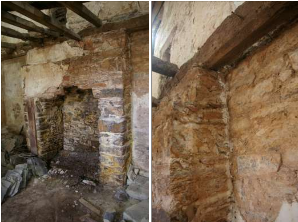
63. (LEFT) DETAIL OF FIREPLACE FP2, SHOWING ITS ABUTTING AND PARTIALLY FORCED RELATIONSHIP WITH THE NORTH-EAST WALL OF B1; VIEWED FROM THE SOUTH.
