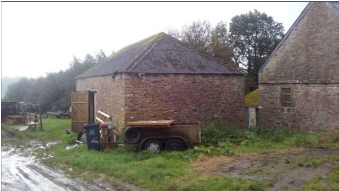
95. DETAIL OF THE NORTH-WESTERN CORNER OF THE NORTH-EAST AND NORTH-WEST ELEVATIONS OF B2; VIEWED FROM THE NORTH.
