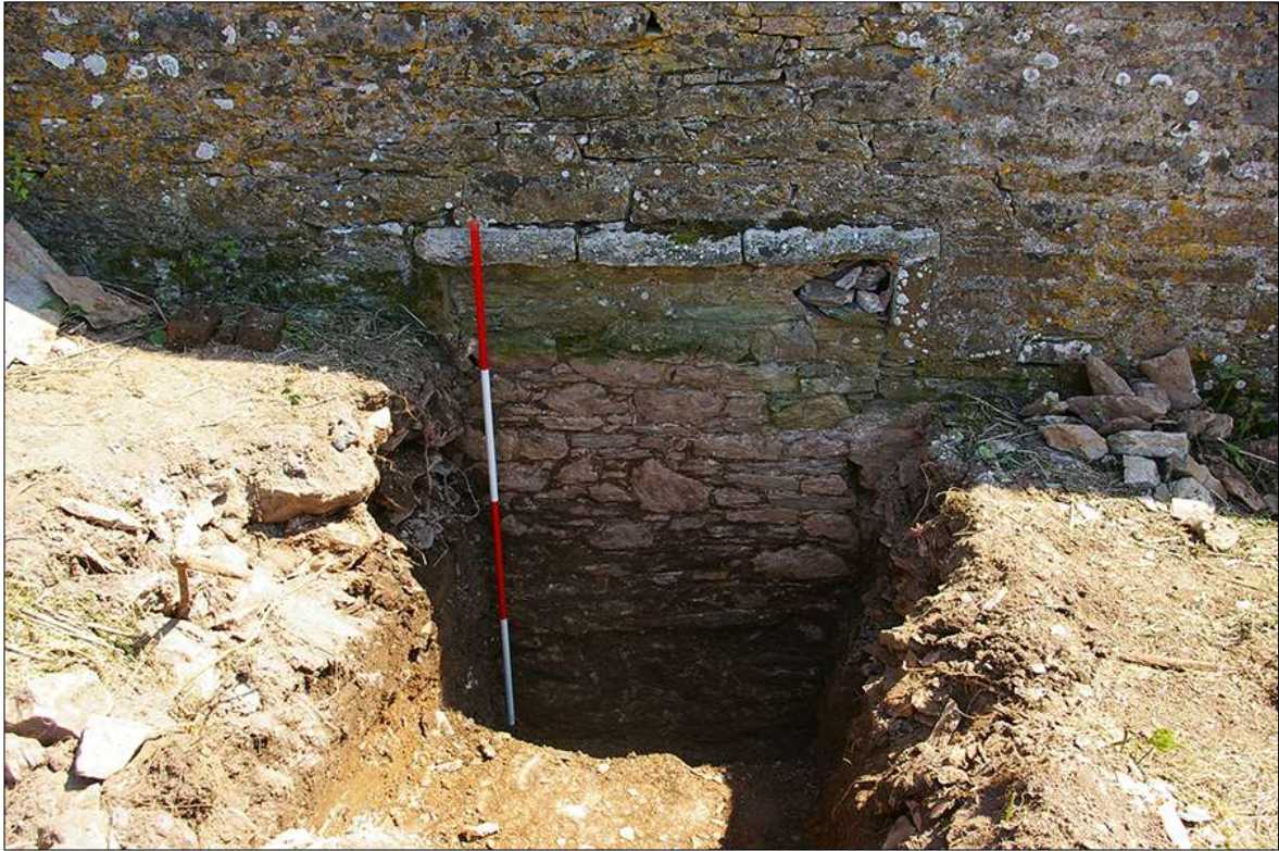
16. DETAIL OF THE BLOCKED AND PARTIALLY BURIED W3 WITHIN THE NORTH-WEST ELEVATION OF B1; VIEWED FROM THE NORTH-WEST (2M SCALE).
