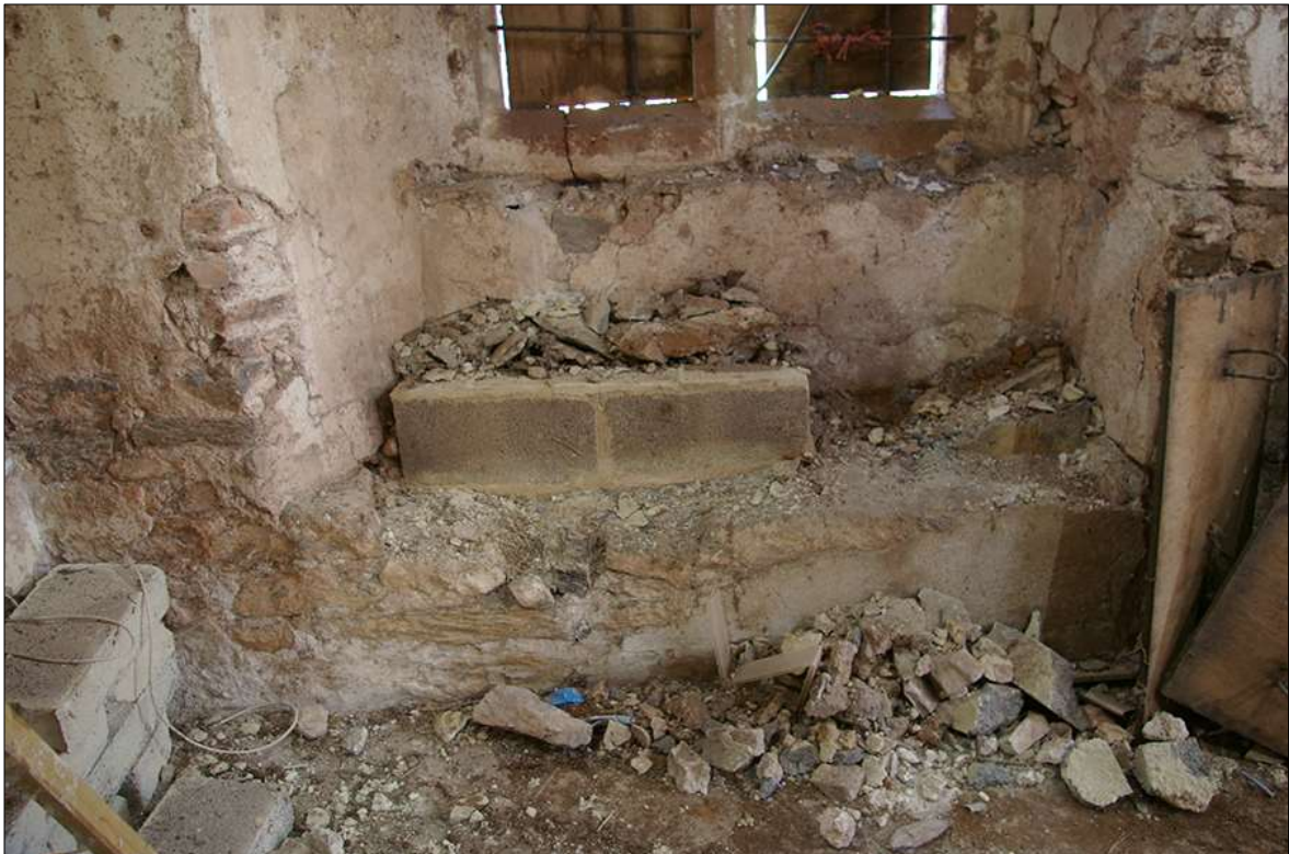
70. DETAIL OF THE HEAVY SLAB INFILL BELOW WINDOW W7, SET INTO THE BLOCKED DOORWAY; VIEWED FROM THE NORTH-WEST.
