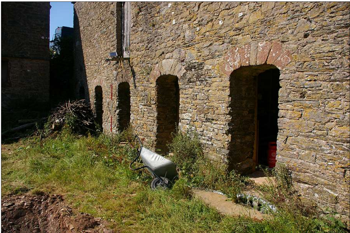
90. DETAIL OF THE SOUTH-WEST ELEVATION OF B2 SHOWING THE FIVE ANIMAL HOUSING OPENINGS; VIEWED FROM THE SOUTH (2M SCALE).
