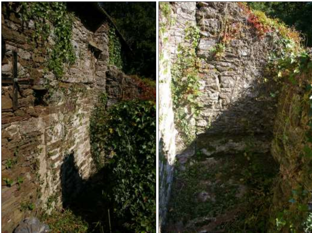
103. (LEFT) DETAIL OF BLOCKED DOOR D11 TO THE 'GARDEROBE' THROUGH THE SOUTH-WEST ELEVATION OF B3; VIEWED FROM THE WEST.
