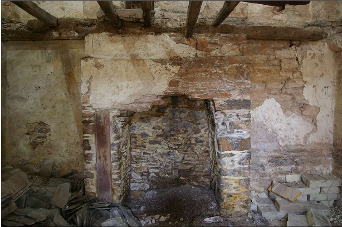
62. DETAIL OF FIREPLACE FP2 IN THE NORTH-EAST WALL OF THE NORTH-EAST ROOM OF B1, SHOWING RAGGED PATCHED SIDES AND EXTENSION OF THE STACKS JAMBS OUTWARDS; VIEWED FROM THE SOUTH-WEST.
