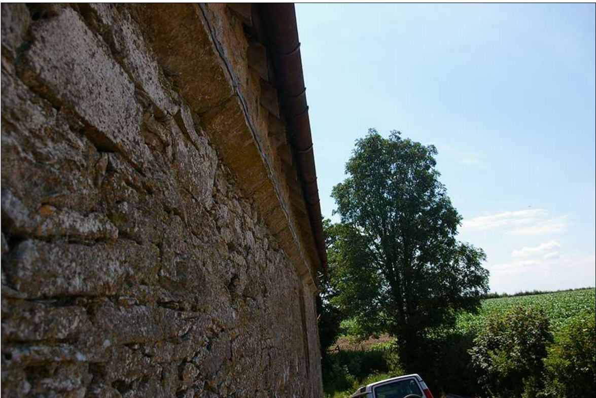
11. DETAIL OF THE FINE DRESSED CHAMFERED EAVES CORNICE ON THE NORTH-WEST ELEVATION OF B1; VIEWED FROM THE NORTH.
