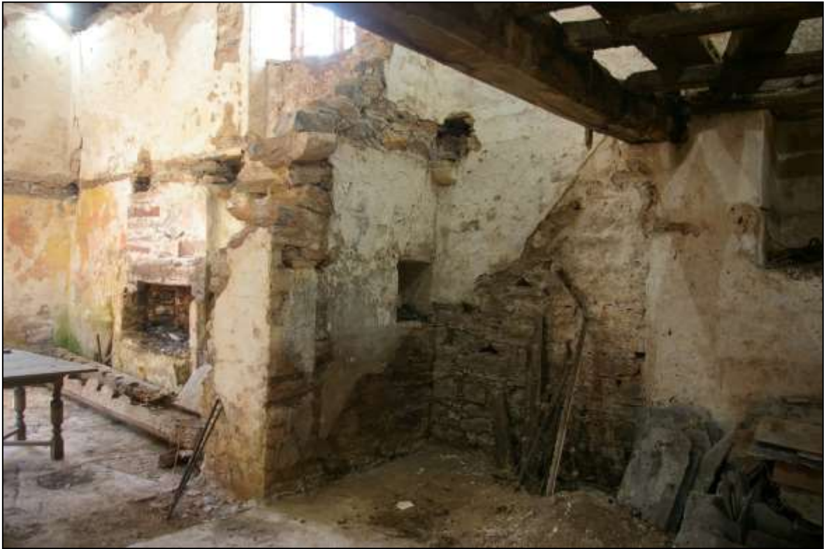
FIGURE 8: DETAIL OF THE INTERIOR OF B1, SHOWING THE SCAR OF THE REMOVED STAIRS TO THE FIRST FLOOR; VIEWED FROM THE SOUTH-EAST.
