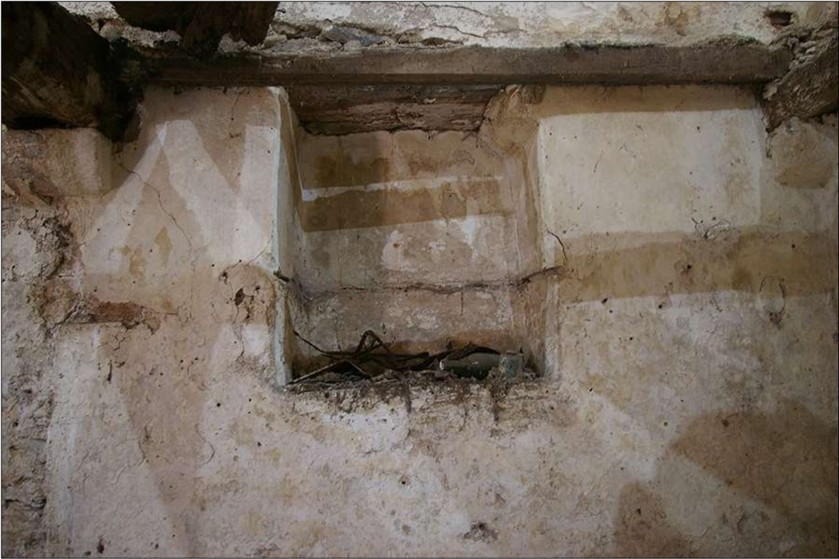
67. DETAIL OF THE ALCOVE SET IN THE NORTH-WEST WALL OF B1, NOTE THE SCAR FOR A SMALL SHELF; VIEWED FROM THE SOUTH-EAST.
