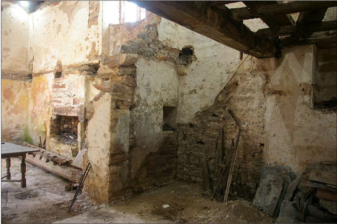
71. DETAIL OF CROSS-WALL BETWEEN THE TWO GROUND-FLOOR ROOMS OF B1; VIEWED FROM THE EAST.
