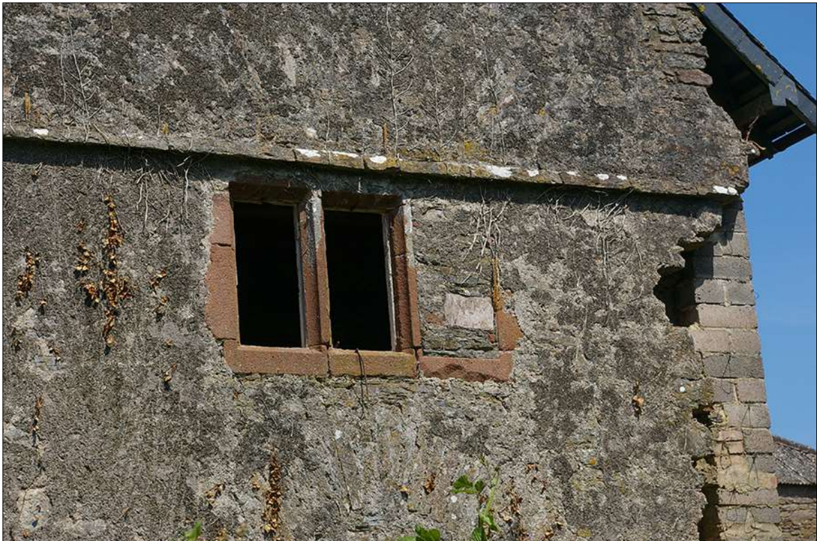
21. DETAIL OF WINDOW W6 IN THE SOUTH-WEST ELEVATION OF B1, DEMONSTRATING THE SINGLE BLOCKED LIGHT; VIEWED FROM THE SOUTH-WEST.
