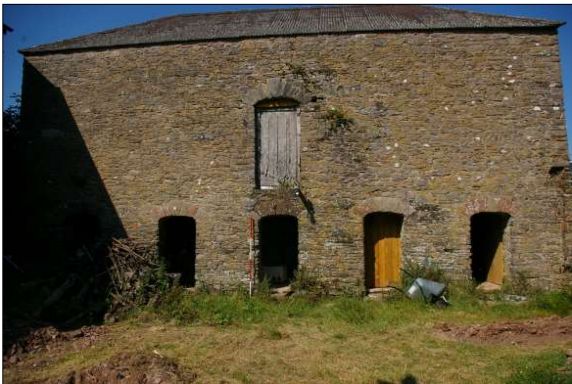
FIGURE 9: BANK BARN B2, SHOWING THE MULTIPLE PHASES OF ALTERATION WITHIN THE SOUTH-WEST ELEVATION; VIEWED FROM THE SOUTH-WEST (2M SCALE).
