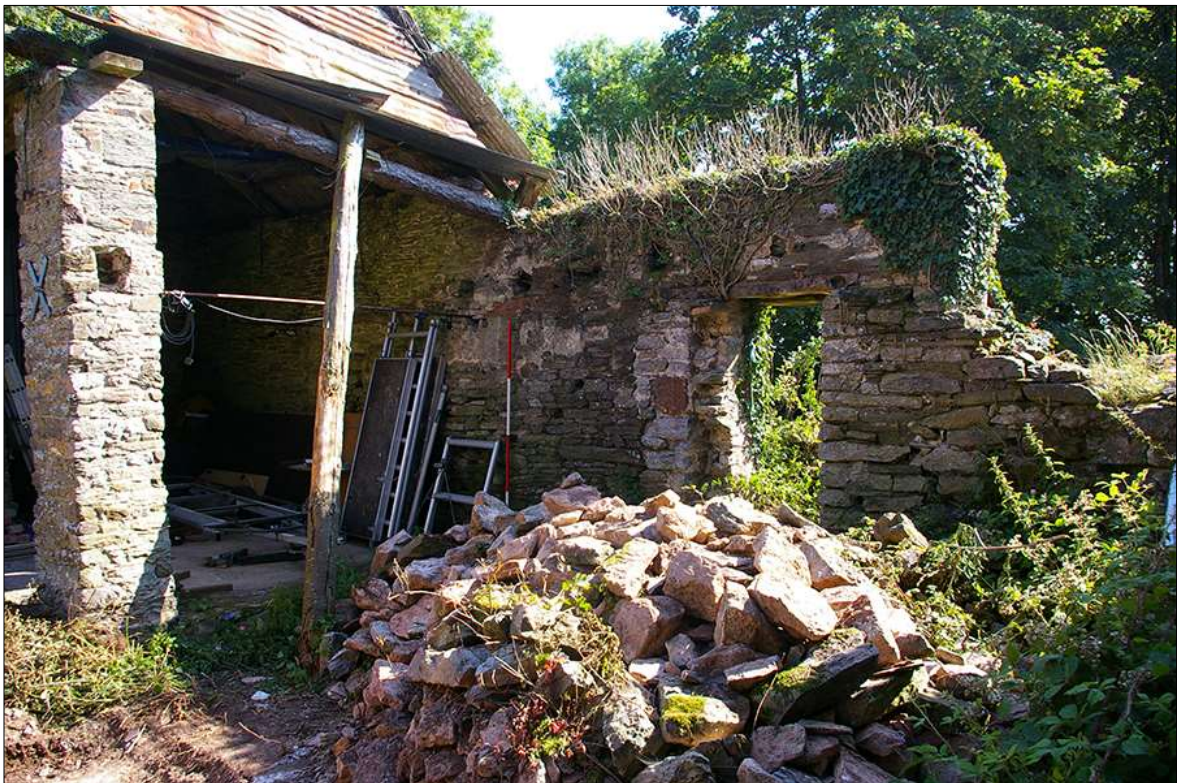
112. INTERIOR FACE OF THE SOUTH-WEST ELEVATION (NORTH-WEST END) OF B3; VIEWED FROM THE EAST (2M SCALE).
