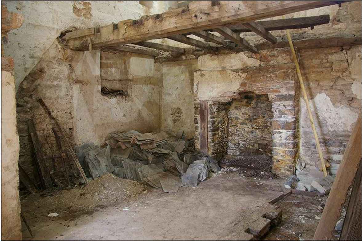
58. THE SMALLER NORTH-EAST GROUND-FLOOR ROOM WITHIN B1, SHOWING LARGE FIREPLACE FP2; VIEWED FROM THE SOUTH.
