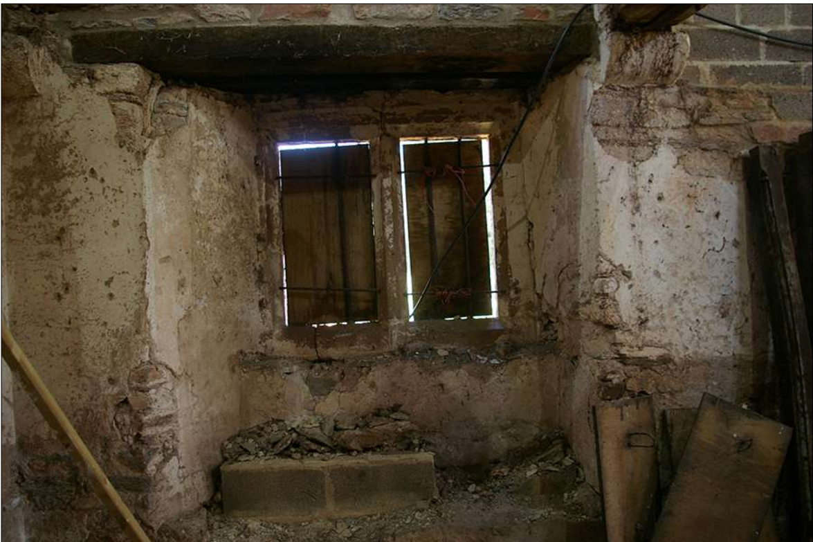
68. WINDOW W7 SET WITHIN THE EARLIER BLOCKED DOORWAY IN THE SOUTH-EAST WALL OF B1; VIEWED FROM THE NORTH-WEST.
