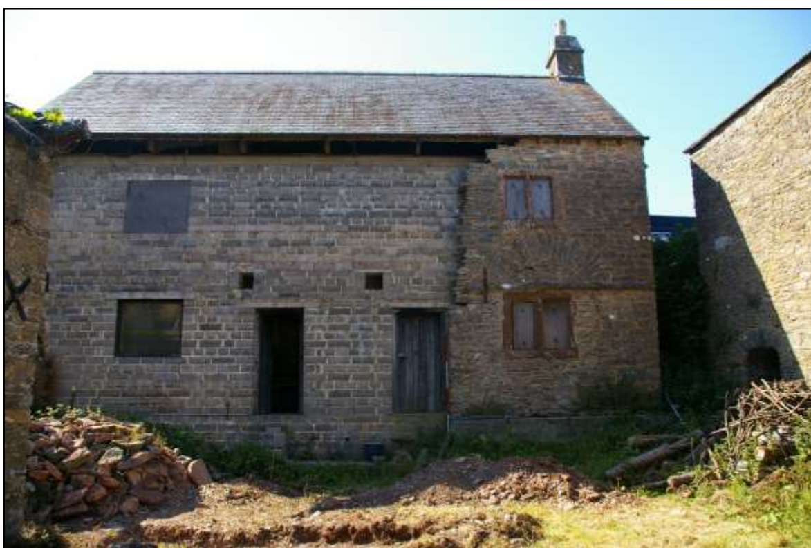
FIGURE 3: THE SOUTH-EAST ELEVATION OF B1 SHOWING THE EXTENSIVE MODERN REPAIRS; VIEWED FROM THE SOUTH-EAST (2M SCALE).
