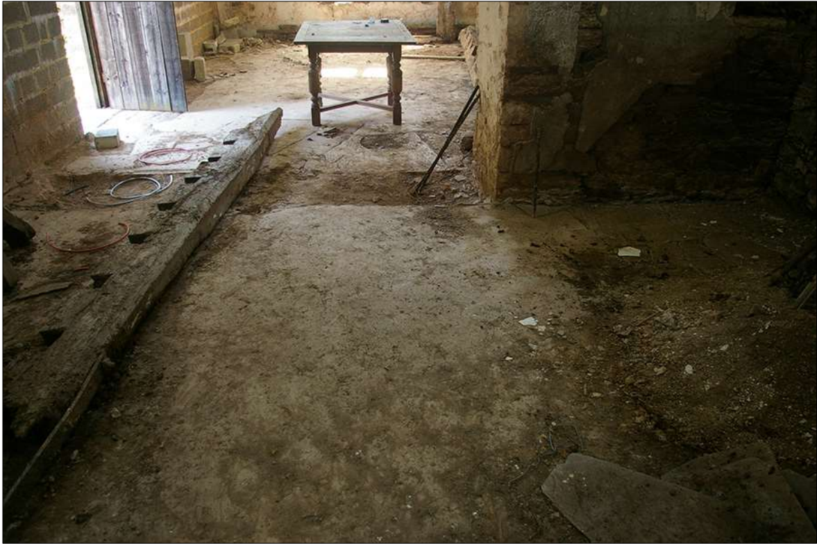
60. DETAIL OF THE CONCRETE FLOOR TO THE NORTH-EAST GROUND-FLOOR ROOM WITHIN B1; VIEWED FROM THE NORTH-EAST.
