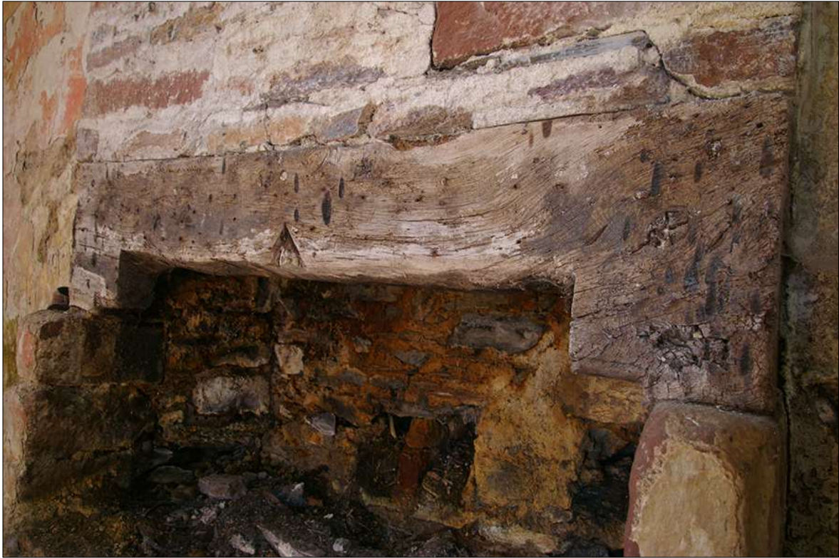
48. DETAIL OF THE RE-USED TIMBER LINTEL OF FIREPLACE FP1, WITH CUT OFF OVULO MOULDING AND TRUNCATED CENTRAL MULLION SUGGESTING THAT IT IS FROM A TWO-LIGHT WINDOW; VIEWED FROM THE EAST.
