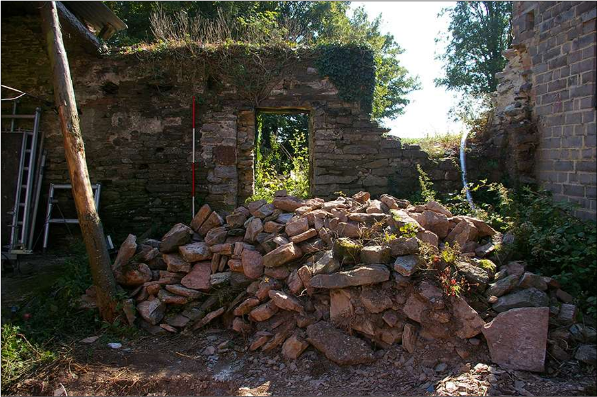
113. INTERIOR FACE OF THE SOUTH-WEST ELEVATION (NORTH-WEST END) OF B3 SHOWING THE EXTENT OF STORM DAMAGE; VIEWED FROM THE NORTH-EAST.
