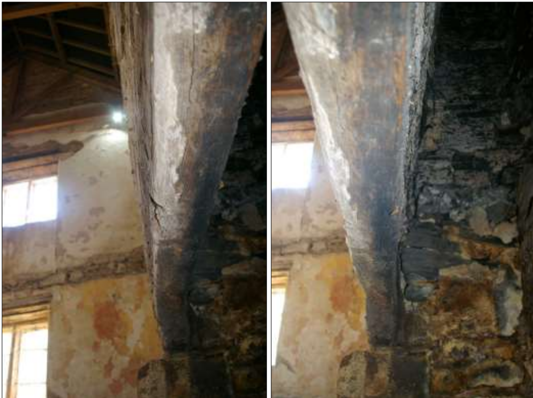
49. (LEFT) DETAIL OF RE-USED TIMBER LINTEL OVER FIREPLACE FP1; VIEWED FROM THE NORTH-EAST.
