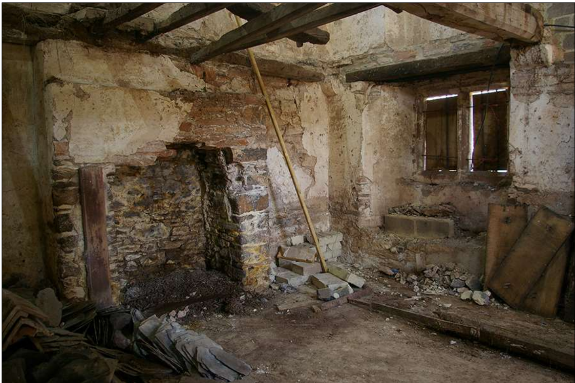
59. THE SMALLER NORTH-EAST GROUND-FLOOR ROOM WITHIN B1, SHOWING LARGE FIREPLACE FP2 AND WINDOW W7; VIEWED FROM THE WEST.
