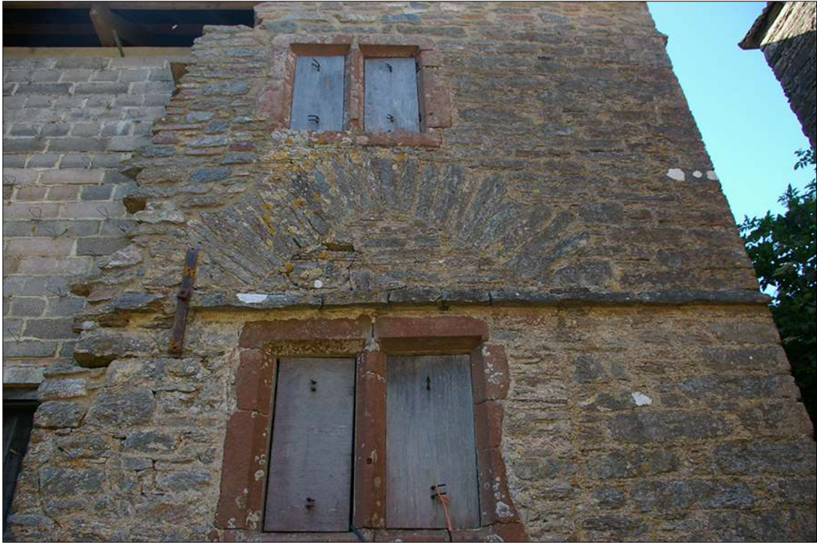
26. DETAIL OF THE THIN SLATESTONE SLAB POINTED SEGMENTAL ARCH OVER BLOCKED DOORWAY (NOW WINDOW) W7; VIEWED FROM THE SOUTH-EAST.
