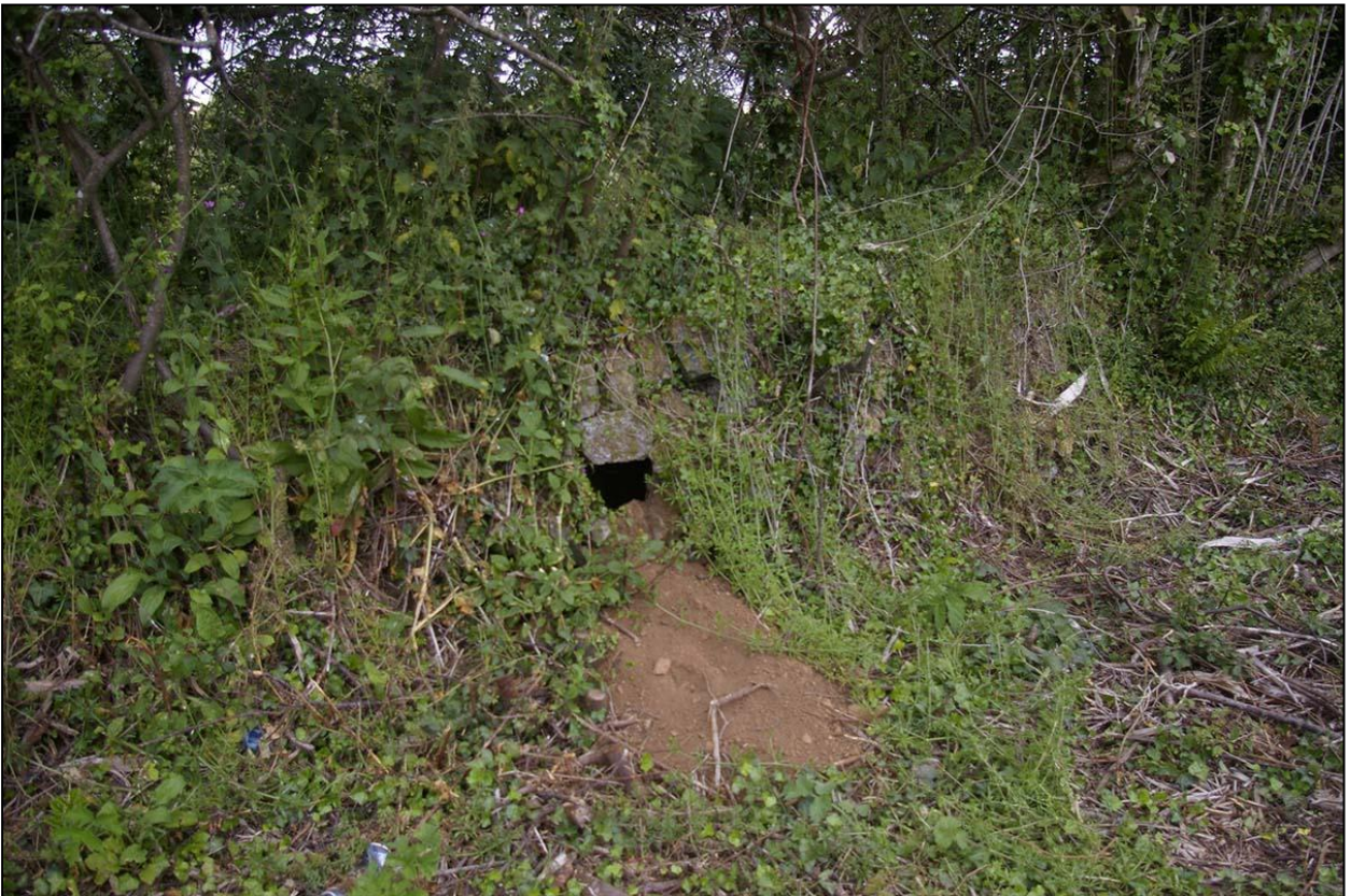
DETAIL OF THE WEST SITE BOUNDARY SHOWING BADGER SETT DAMAGE; VIEWED FROM THE SOUTH.
