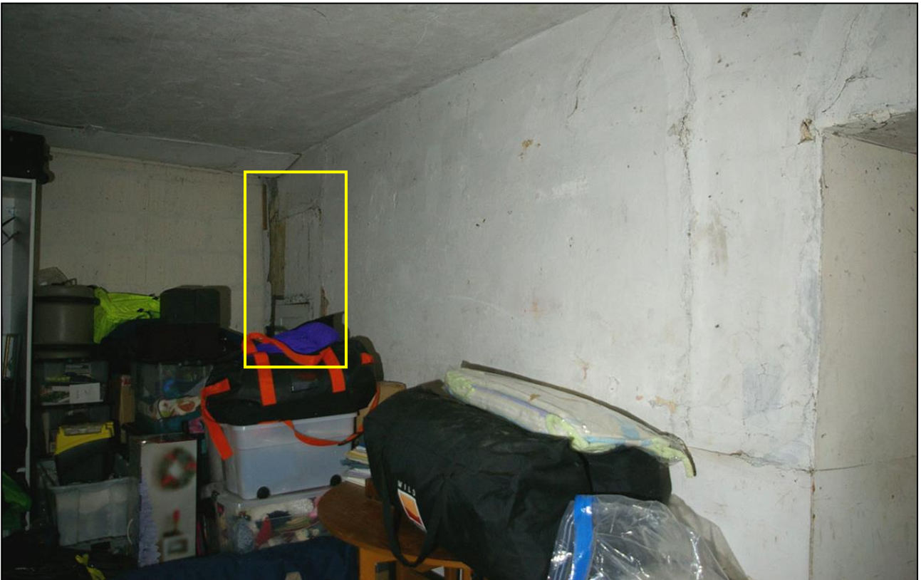
R3, THE HEAVY BATTERED FORMER GABLE END WALL OF THE 17 TH CENTURY BUILDING, SHOWING ORIGINAL DOOR TO THE NORTH END (INDICATED), NOW FITTED AS A CUPBOARD; VIEWED FROM THE SOUTH-SOUTH-WEST.
