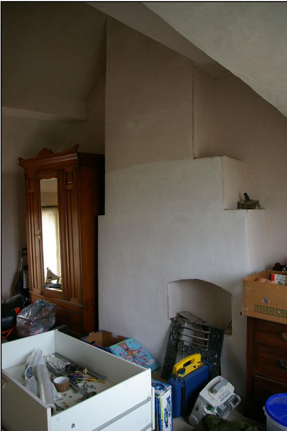
R15, THE BRICK STACK, BUILT UP AGAINST THE WALL OF THE OLD BAKEHOUSE; VIEWED FROM THE NORTH-EAST.
