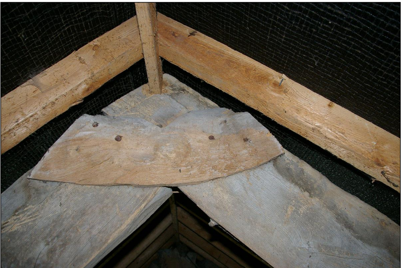
R17, DETAIL OF ONE OF THE RIDGES, WITH SPIKED YOKES BRACING THE OVERLAPPING RIDGE JOINT, ALSO CUT WITH A DIAMOND SET FOR A RIDGE POLE, ALTHOUGH REPLACED, AS THE ROOF HAS BEEN ALTERED; VIEWED FROM THE WEST.
