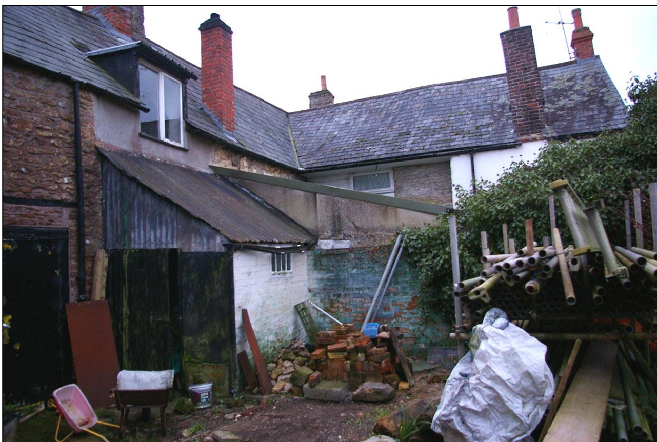
THE SMALL 19 TH CENTURY BRICK SHED BUILT UP AGAINST THE RENDERED CONCRETE BLOCK INFILL THAT LINKS THE TWO BUILDINGS; VIEWED FROM THE EAST-NORTH-EAST.
