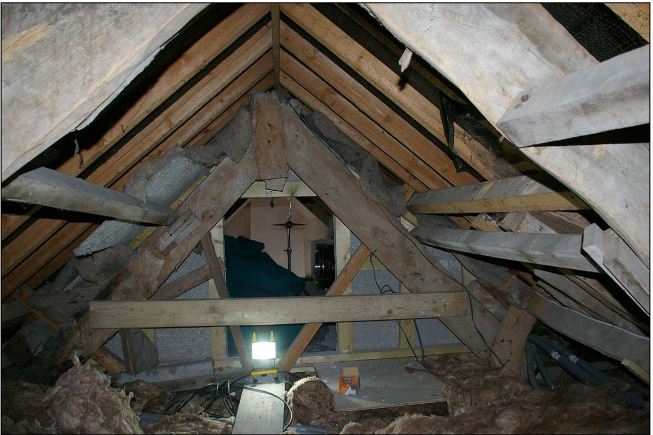
R17, VIEW BACK TO THE TRUSS BETWEEN R16 AND R17; VIEWED FROM THE EAST.
