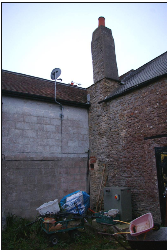
THE LATERAL STACK AND ADJACENT REDUCED OPENING ON THE NORTH WALL OF ASH HOUSE; VIEWED FROM THE NORTH-WEST.
