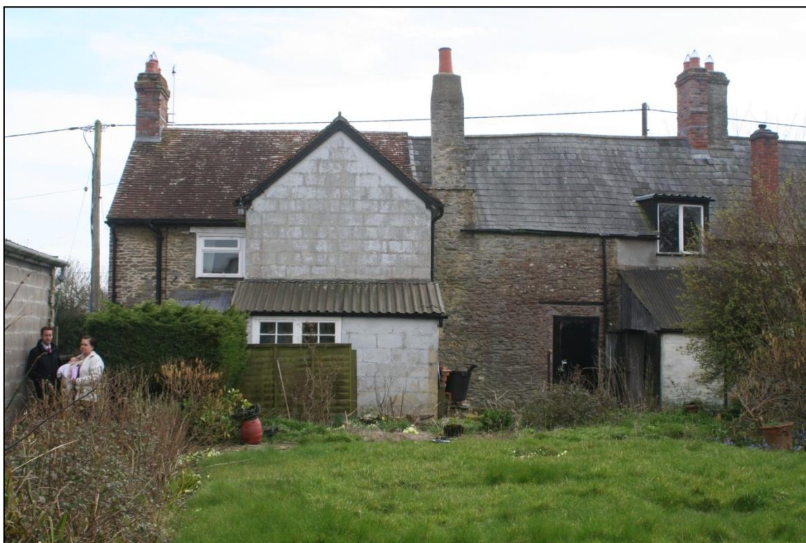
FIGURE 8: THE NORTH ELEVATION OF THE COTTAGE WEST OF THE REAR EXTENSION; VIEWED FROM THE NORTH.
