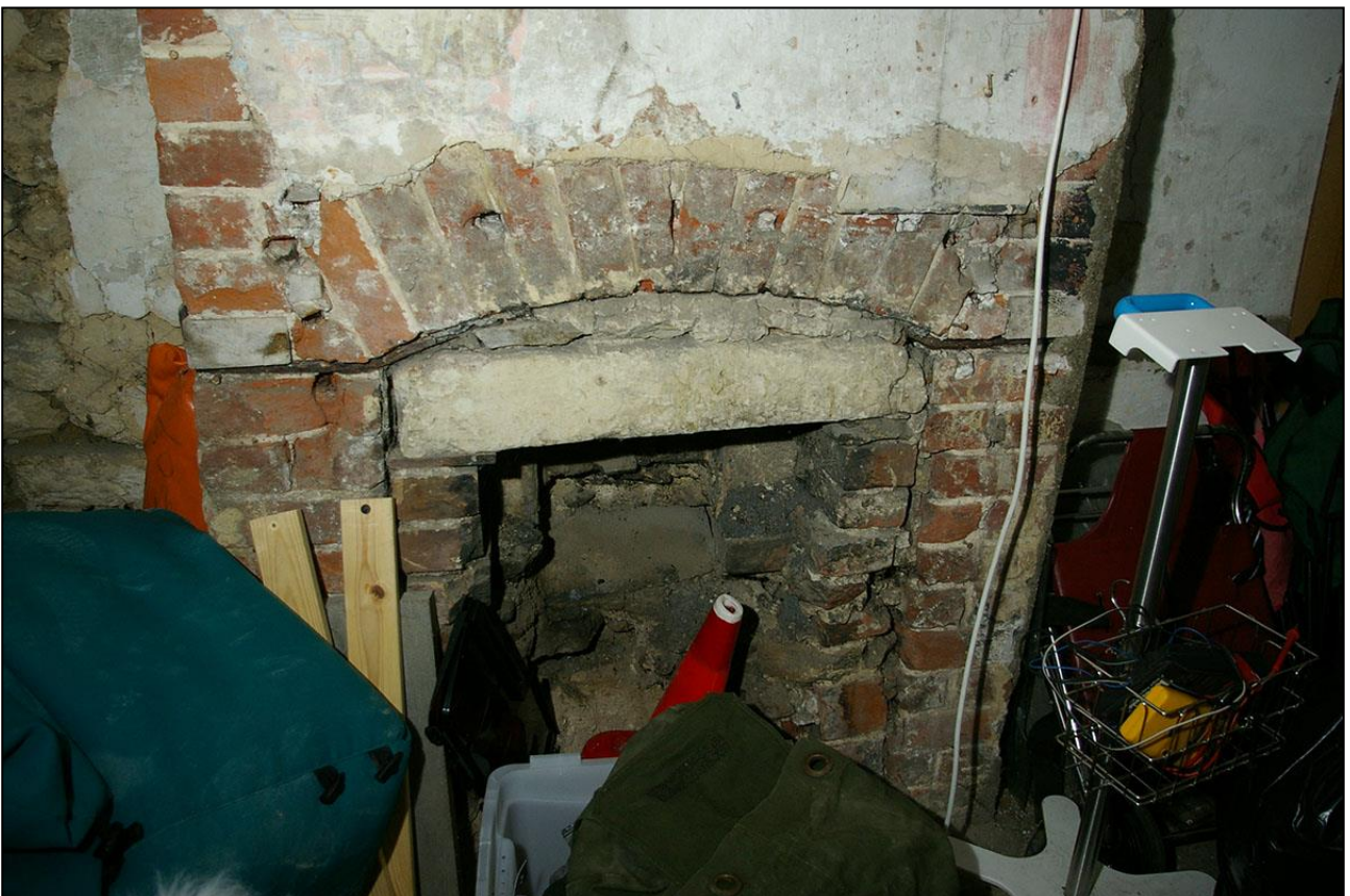
R3, DETAIL OF THE BRICK STACK SHOWING THE LARGE BOX HEARTH WITH SEGMENTAL BRICK ARCH AND IRON BAR SUPPORT, WITH LATER INFILL; VIEWED FROM THE SOUTH-EAST.
