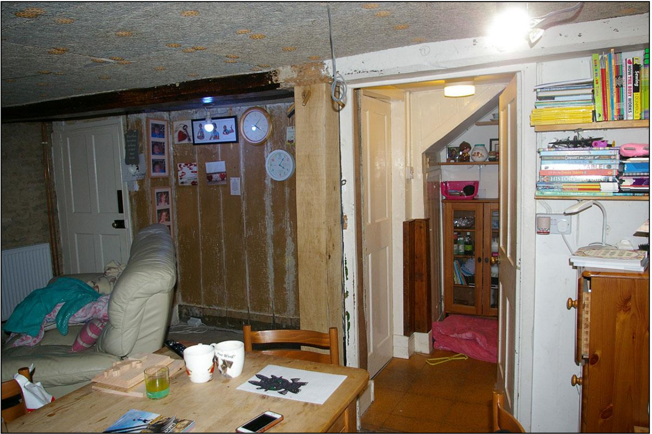
R4, THE TIMBER PARTITION WALL ENCLOSING THE STAIRS (LEFT), WITH DOORS TO R1 AND R5; VIEWED FROM THE NORTH-EAST.
