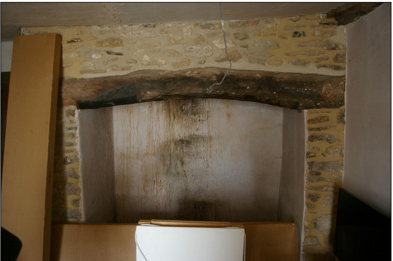
R2, THE FIREPLACE, NEWLY REPOINTED AND PLASTERED, THE LARGE BRESUMMER BEAM HACKED ON THE UNDERSIDE; VIEWED FROM THE SOUTH.
