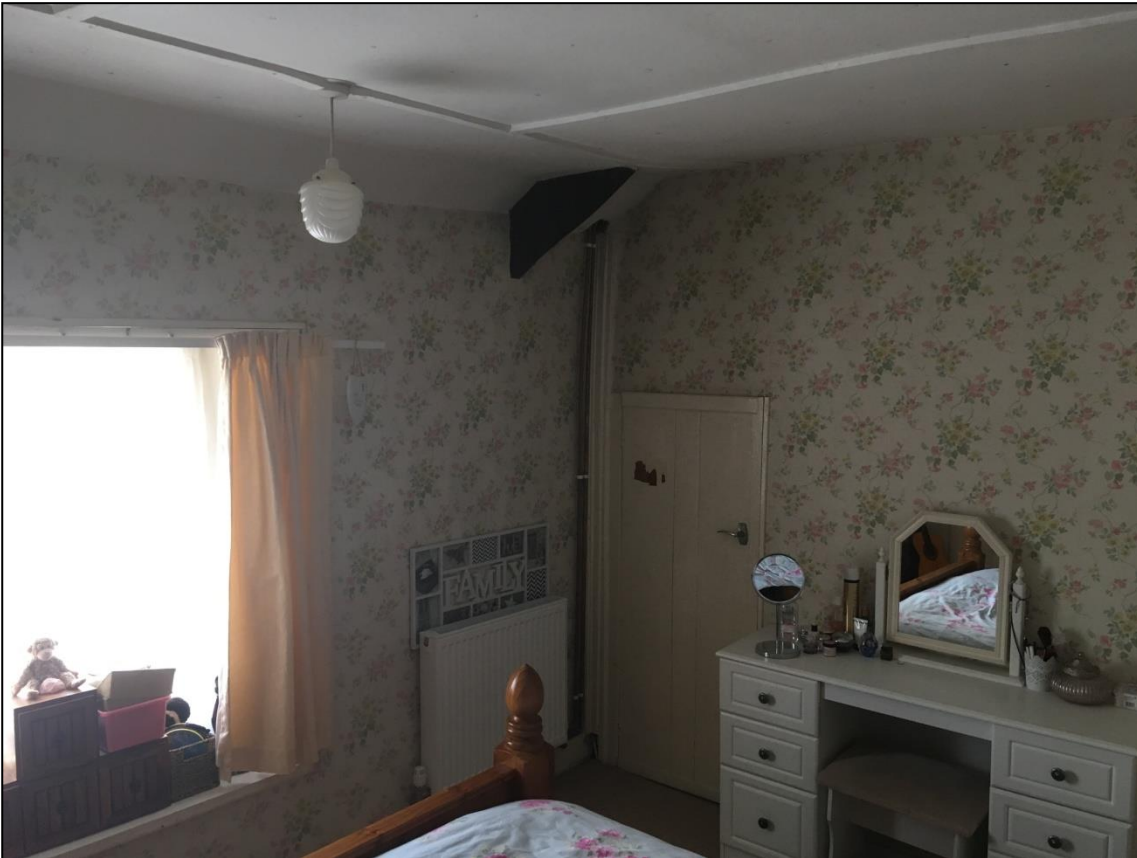
R11, SHOWING THE LOW PLANK DOOR (LEFT) TO THE DEEP CUPBOARD THAT FORMERLY PROVIDED ACCESS TO R10; VIEWED FROM THE NORTH-EAST (SUPPLIED BY CLIENT).
