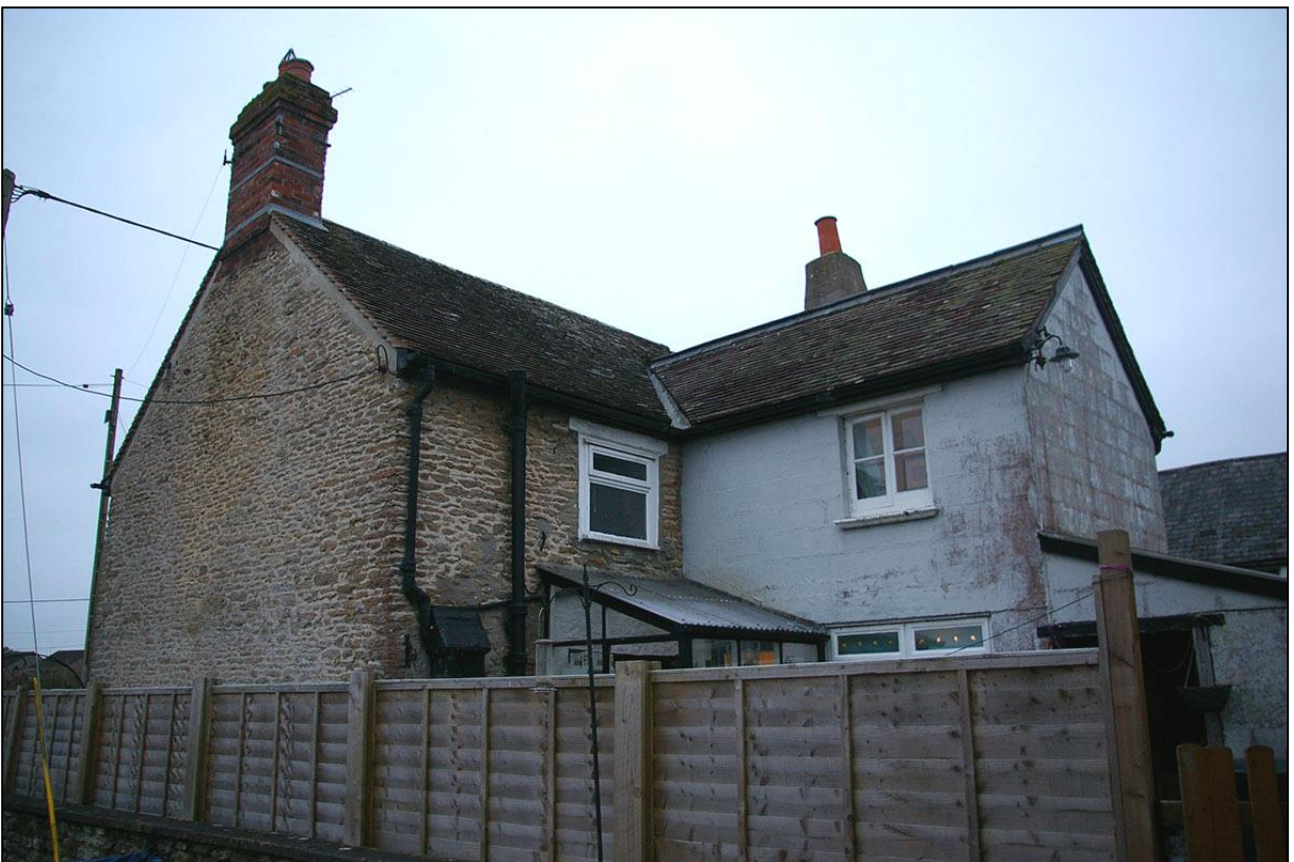
ASH HOUSE AND ITS 20 TH CENTURY CONCRETE BLOCK KITCHEN EXTENSION; VIEWED FROM THE NORTH-EAST.
