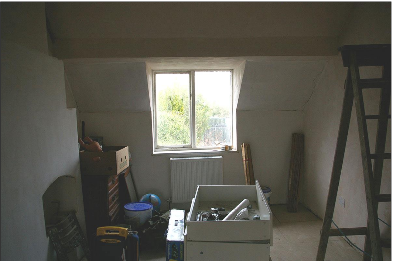
R15, THE NORTH WALL WITH MID 20 TH CENTURY WINDOW IN LOW WALL; VIEWED FROM THE SOUTH.
