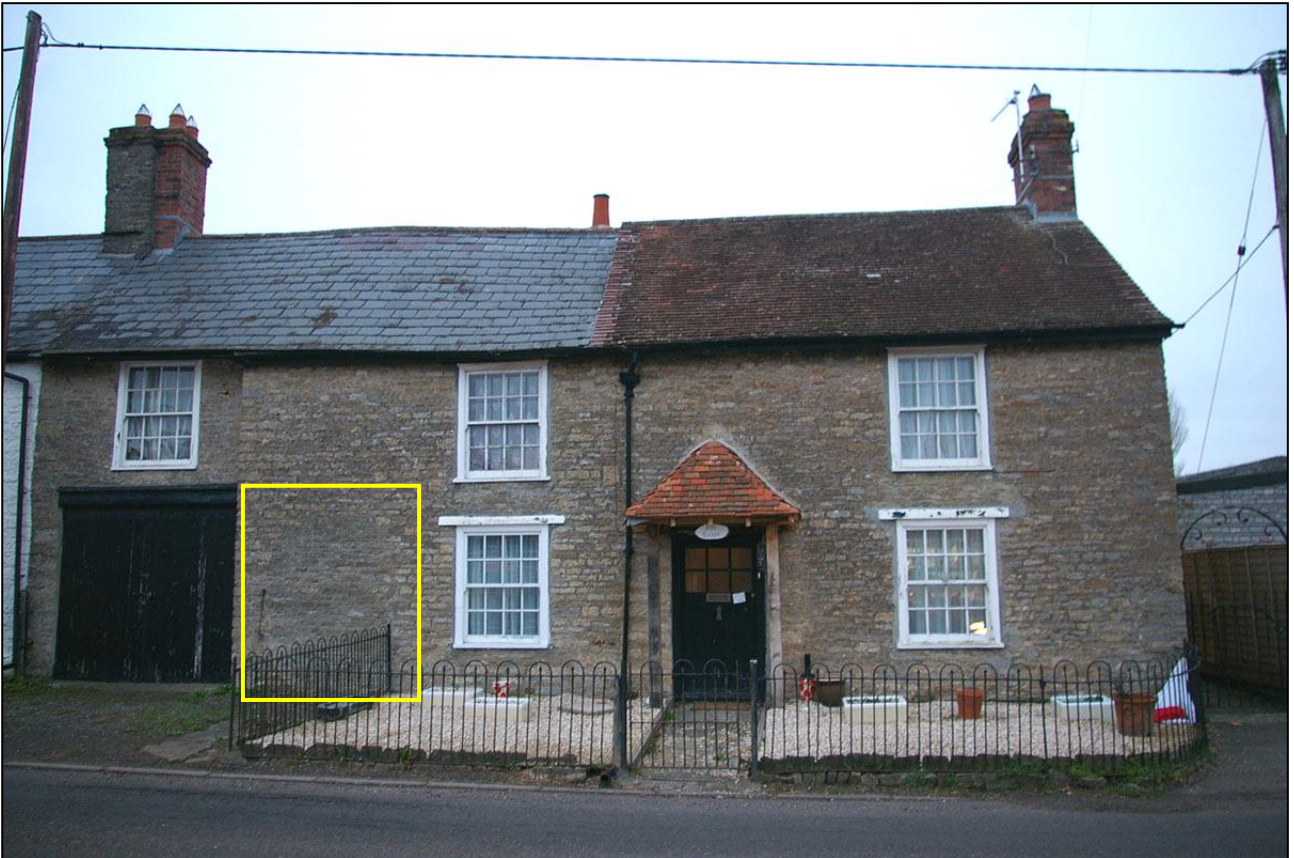
THE SOUTH ELEVATION OF ASH HOUSE, SHOWING A BLOCKED DOOR OPENING TO THE WEST END (INDICATED); VIEWED FROM THE SOUTH-SOUTH-EAST.
