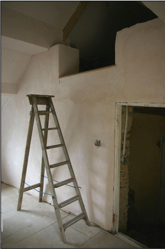
R15, THE FORMER GABLE END WALL OF THE ORIGINAL COTTAGE, FORCED TO PROVIDE WIDER ACCESS TO THE LOFT SPACE ADJACENT; FROM THE SOUTH-WEST.
