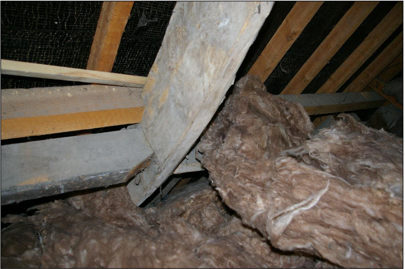
R17, THE HEAVY SQUARE PROFILE PURLINS, AN EARLIER SET OF THROUGH-AND-THROUGH TYPES; VIEWED FROM THE SOUTH-WEST.
