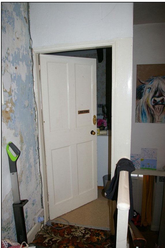
R9, THE 19 TH CENTURY MOULDED FOUR-PANEL DOOR TO R11; VIEWED FROM THE NORTH-WEST.
