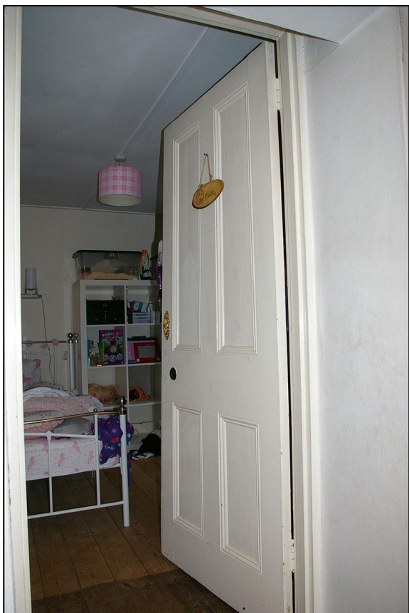
R13, THE FORCED OPENING IN THE BACK WALL PROVIDING ACCESS TO THE 20 TH CENTURY EXTENSION; VIEWED FROM THE SOUTH-SOUTH-WEST.
