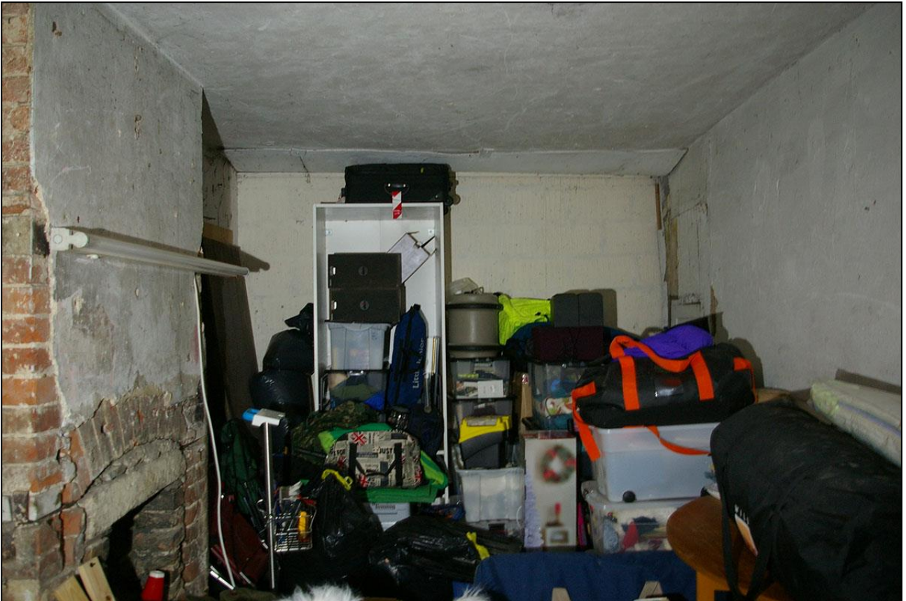
R3, SHOWING THE BRICK STACK BUILT AGAINST THE GABLE WALL OF THE OLD BAKEHOUSE; VIEWED FROM THE SOUTH.
