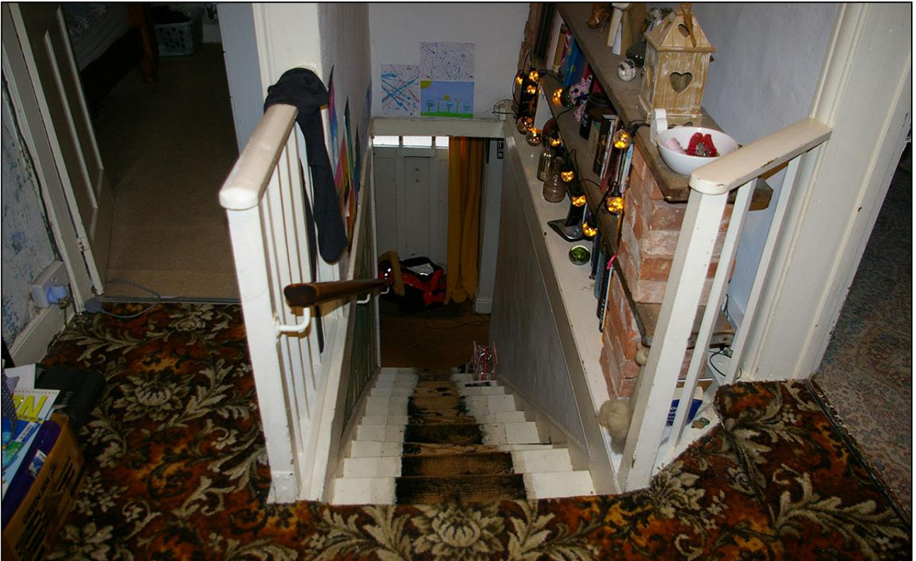
THE TOP OF THE STAIRS (R8) AND LANDING (R9); VIEWED FROM THE NORTH.
