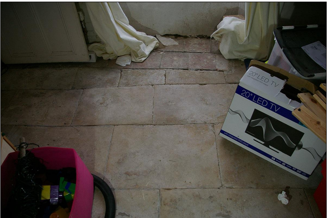
R2, THE FINE STONE FLOOR, WITH STONE AND BRICK PAVERS RESET AGAINST THE FRONT SOUTH WALL SHOWING THE ORIGINAL WIDTH OF THE ROOM, EVIDENCE THAT THE FRONT WALL HAS BEEN REBUILT AND PUSHED OUT; VIEWED FROM THE NORTH.
