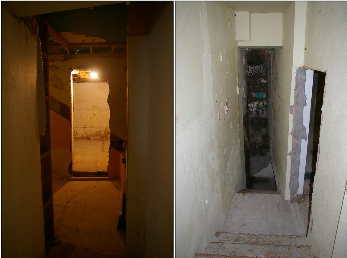
LEFT: VIEW THROUGH VARIOUS FORCED OPENINGS FROM ROOM 2, THROUGH ROOM 3 TO ROOM 4; FROM THE WEST. RIGHT: THE STEEP CONCRETE STEPS LEADING DOWN TO THE DOORWAY TO THE ALLEYWAY, EVIDENCE OF SIGNIFICANT CHANGES IN LEVELS; FROM THE EAST.
