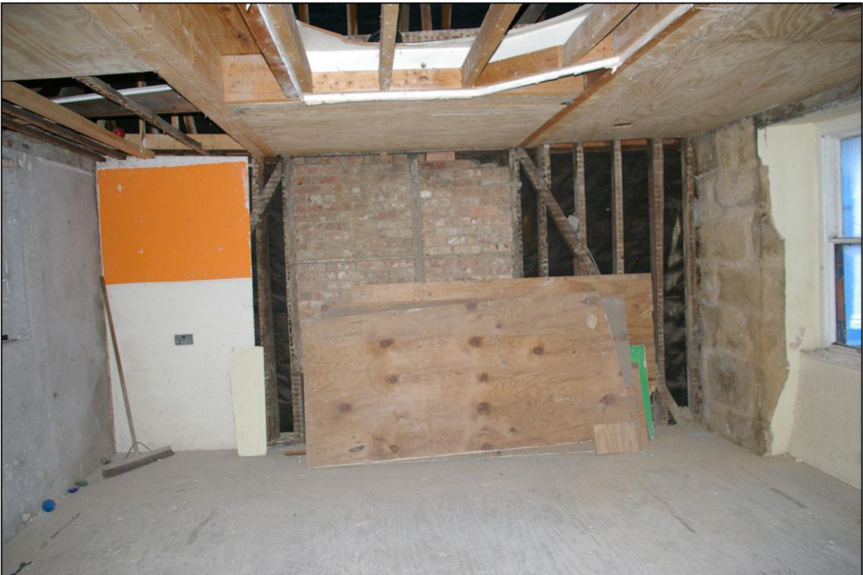
THE STUDWORK SOUTH GABLE END WITH OUTER LAYER OF FELT AND WATERPROOFING AND SMALL SECTION OF BRICK NOGGIN; FROM THE NORTH.
