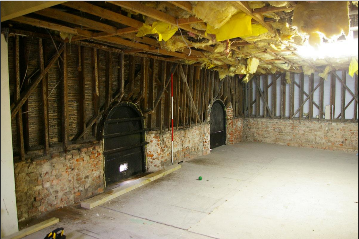
LONG VIEW DOWN THE EAST WALL OF THE SYNAGOGUE, SHOWING THE CLEAR STUDWORK RAISE TO THE BUILDING; FROM THE NORTH-WEST (2M SCALE).
