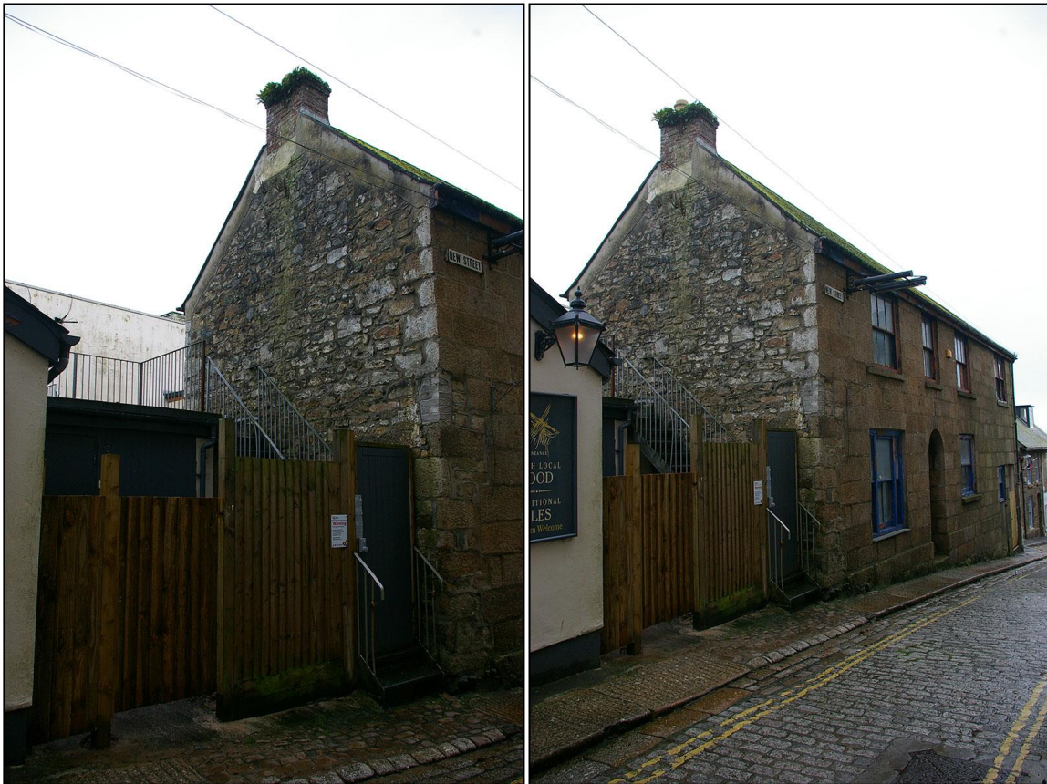
LEFT: THE NORTH GABLE END WALL OF NO.1, A HEAVY GRANITE RUBBLE WALL, WITH ADDED LATER BRICK STACK; FROM THE NORTH-WEST. RIGHT: THE WEST ELEVATION WITH GRANITE ASHLAR RE-FACING, MOST EVIDENT ON THE NORTH-WEST CORNER; FROM THE NORTH-WEST.
