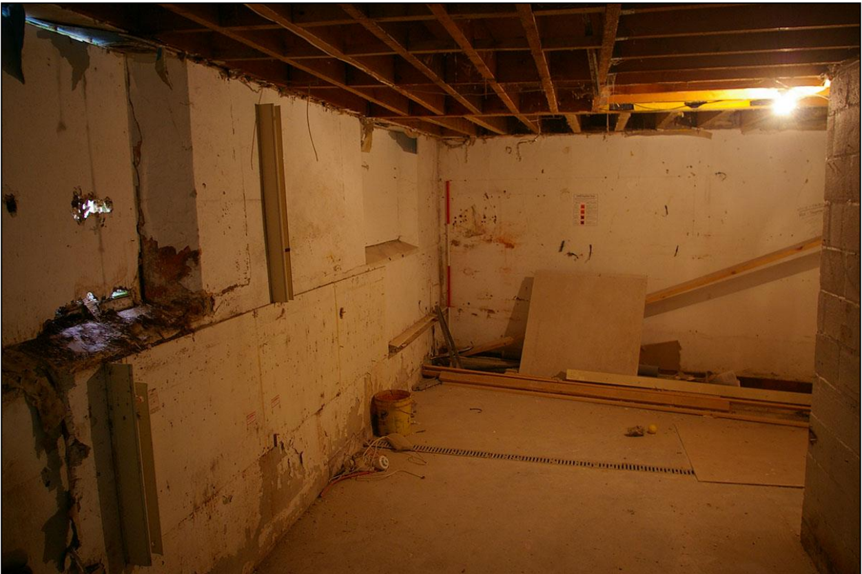
THE EAST AND SOUTH PLASTERED BRICKWORK WALLS OF THE SYNAGOGUE, THE ONLY ELEMENTS WHICH SURVIVE; FROM THE NORTH (2M SCALE).
