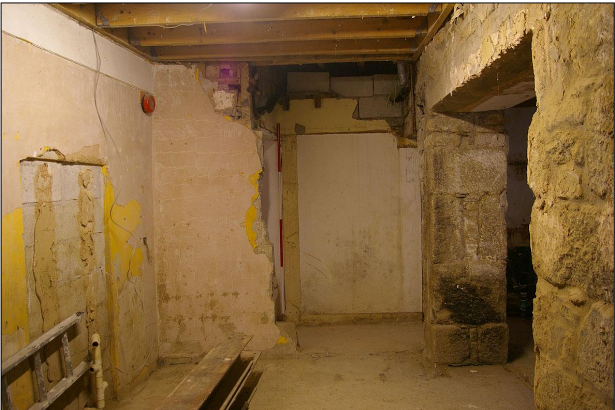
ROOM 2, BEHIND NO.1 NEW STREET, INFILL OF A FORMER OPEN YARD, BUILT OF CONCRETE BLOCK AND BRICK; FROM THE NORTH.
