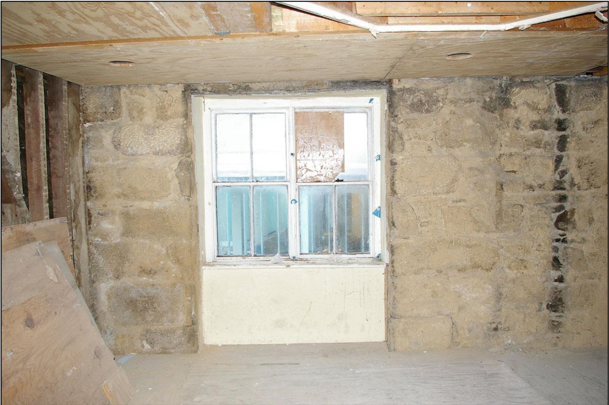
THE DEEP WINDOW ABOVE THE CARRIAGE ARCH IN THE EXTENSION OF NO.1 NEW STREET; FROM THE EAST.
