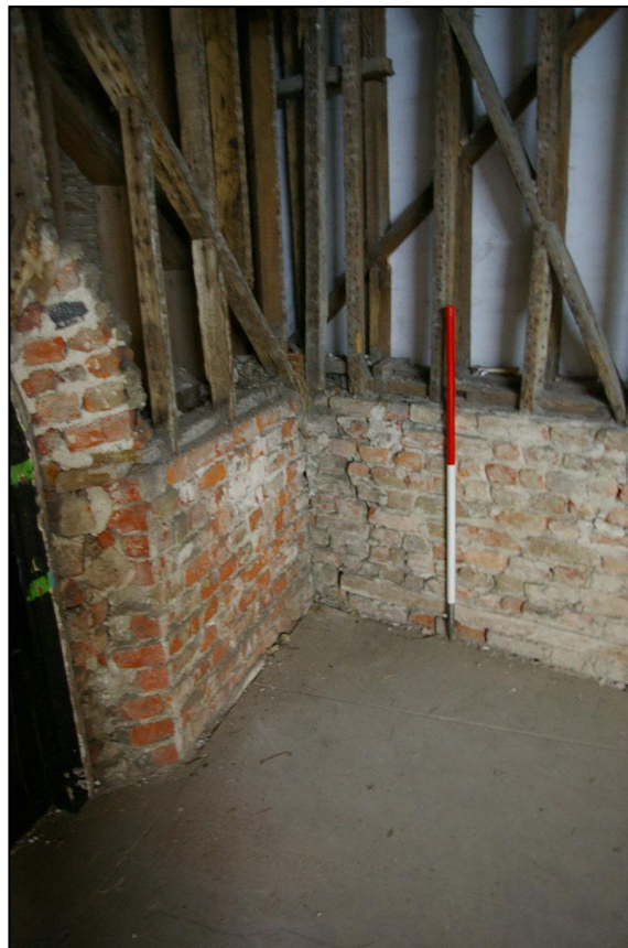
THE SOUTH-EAST CORNER OF THE FORMER SYNAGOGUE, ON THE FIRST FLOOR, ROOM 9, WHERE THE PLASTER HAS BEEN REMOVED, SHOWING DIFFERENT PHASING, THE SOUTH WALL SEEMINGLY ABUTTING THE EAST WALL; FROM THE NORTH (1M SCALE).
