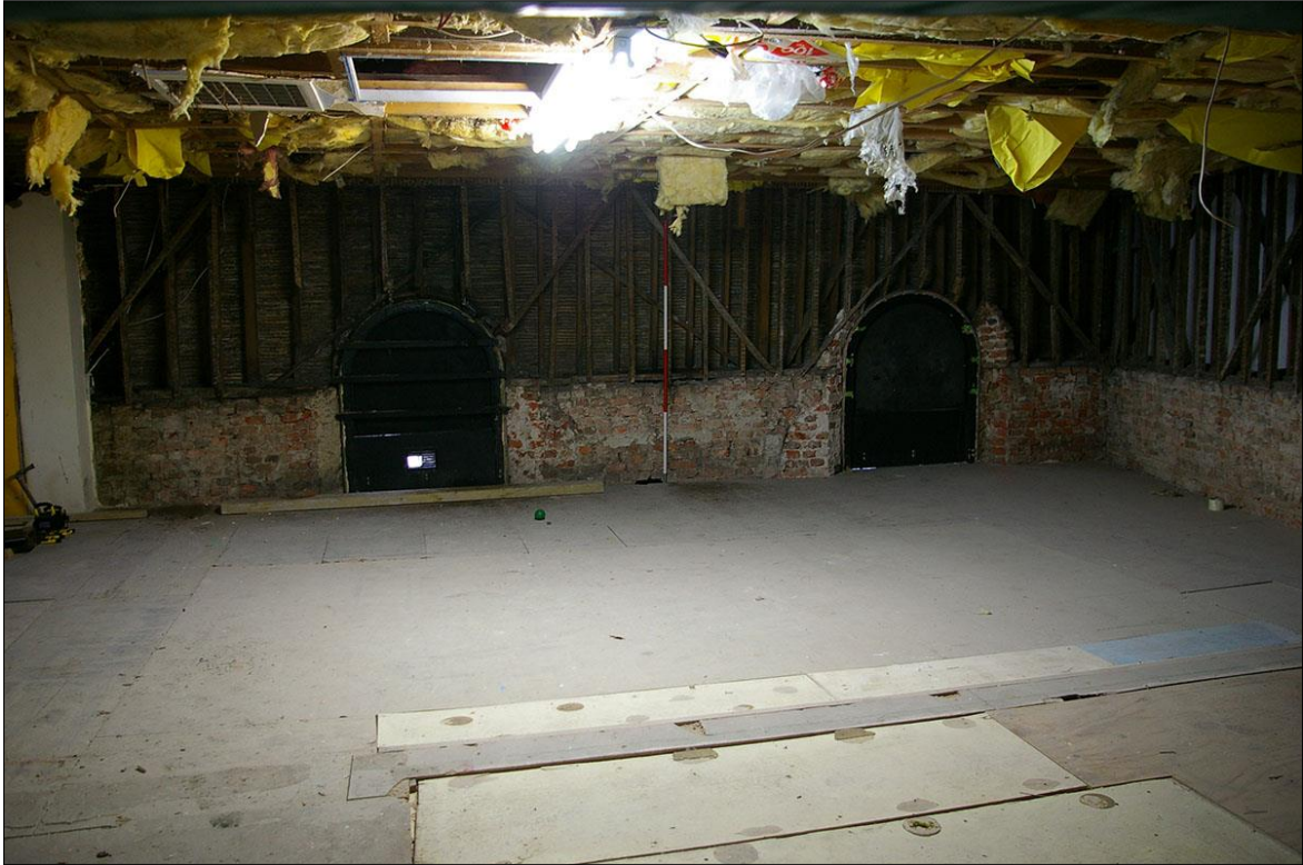
FIGURE 4: THE EAST WALL OF THE SYNAGOGUE, SHOWING THE PHASES OF BRICK AND STUDWORK; FROM THE WEST.
