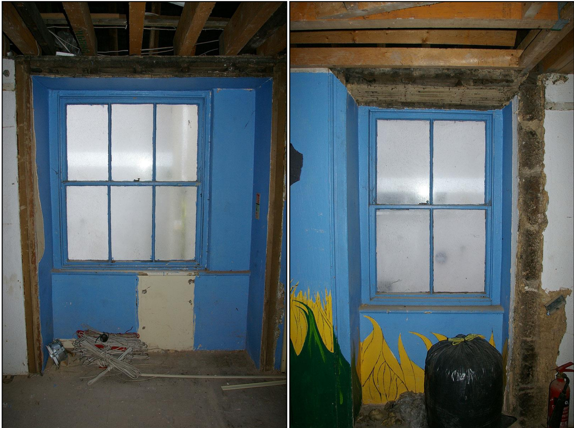
LEFT: ROOM 7, THE WINDOW TO THE NORTH, SET WITHIN A PARTIALLY BLOCKED OPENING, THIS PHASING NOT VISIBLE ON THE ASHLAR FRONTAGE; FROM THE EAST.
