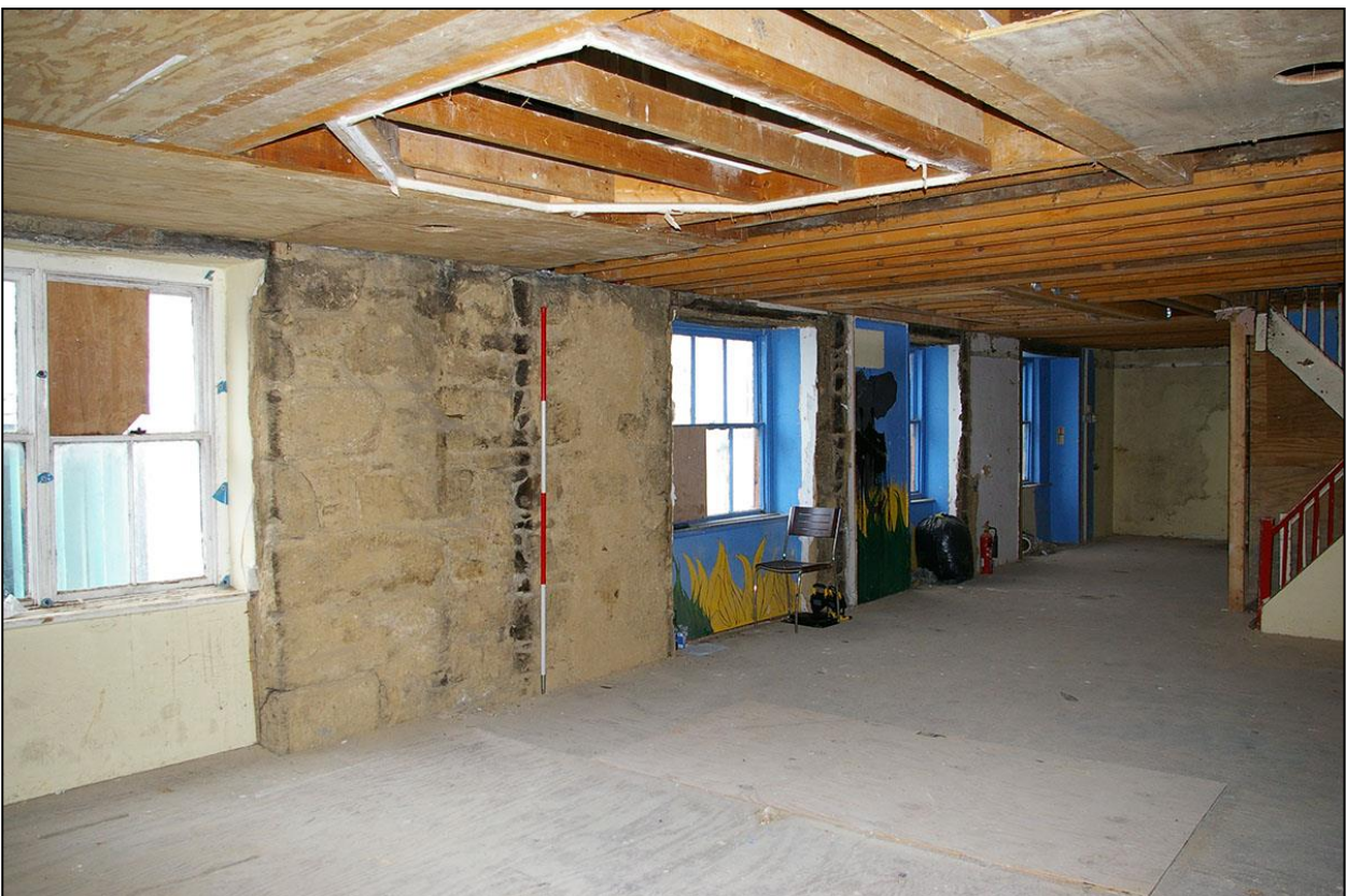
THE WEST WALL OF ROOM 7, SHOWING THE WIDE SECTION OF STONEMWORK ON THE WEST WALL WITH RAGGED BUILD LINE SHOWING WHERE THE BUILDING HAS BEEN EXTENDED; FROM THE SOUTH-EAST (2M SCALE).
