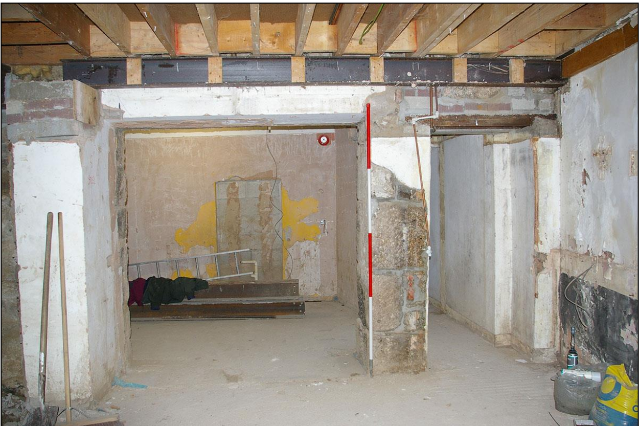
THE ALTERED OPENINGS IN THE REAR WALL OF ROOM 1, NO.1 NEW STREET, THE FORMER ACCESS INTO THE REAR YARD; FROM THE WEST (2M SCALE).
