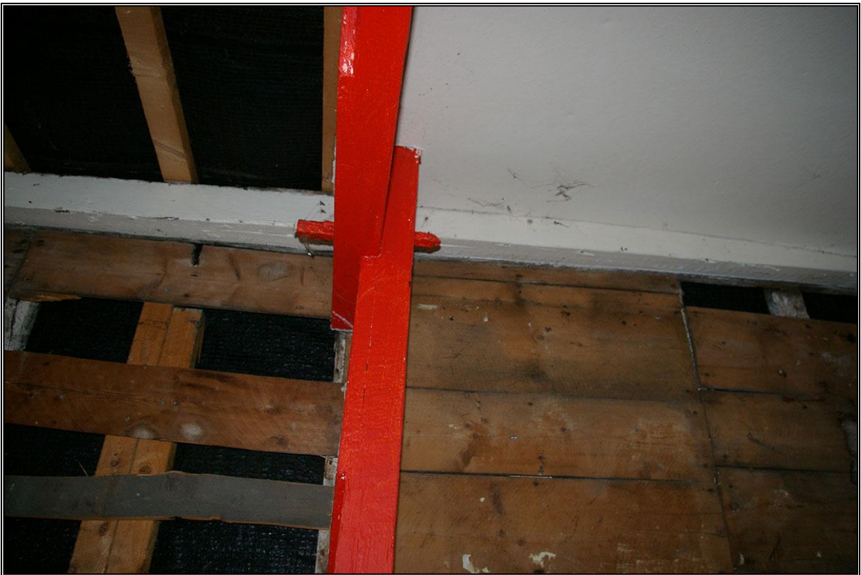
DETAIL OF THE SHALLOW HALF-LAPPING OF THE TRUSS BLADES ON THE PEGGED 18 TH CENTURY TRUSSES TO THE NORTH END OF NO.1 NEW STREET; FROM BELOW.
