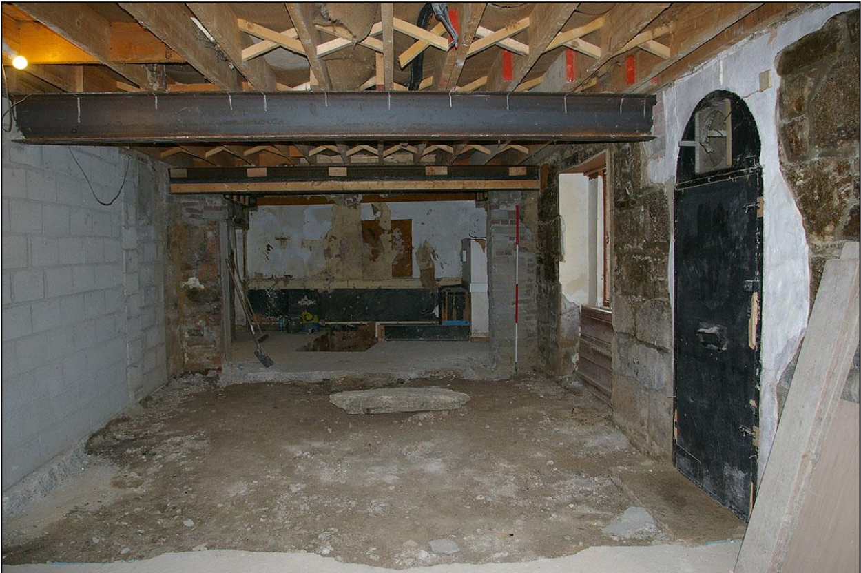
ROOM 6, SHOWING WALLS STRIPPED BACK INDICATING PHASING AND SHOWING TRUNCATED SOUTH GABLE AND CONCRETE FLOOR EXCAVATED; FROM THE NORTH (2M SCALE).
