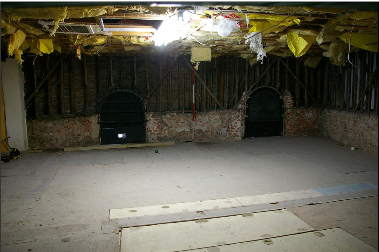
THE EAST WALL OF THE SYNAGOGUE, SHOWING DIFFERENT COLOURS AND BONDS OF BRICKWORK, EVIDENCE OF MUCH ALTERATION IN THE SMALL STRUCTURE; FROM THE WEST (2M SCALE).
