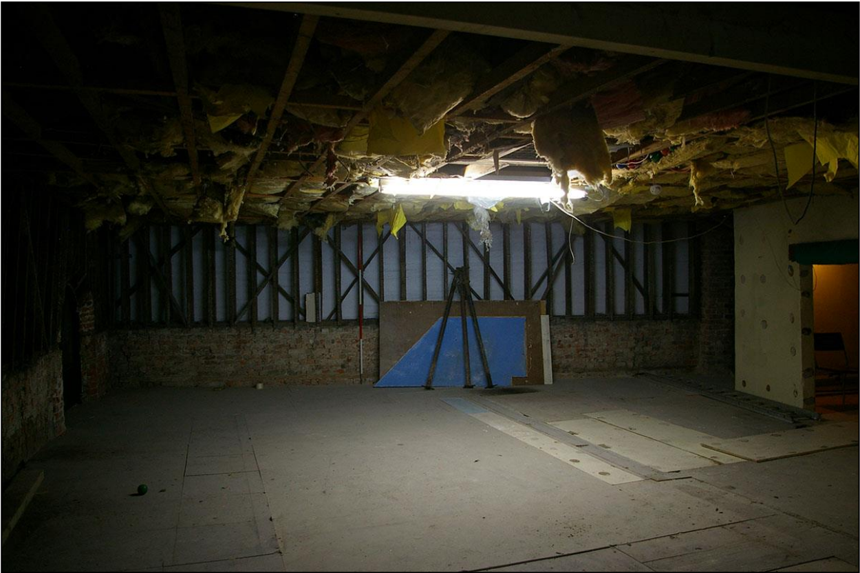
THE ANGLED SOUTH WALL OF THE FORMER SYNAGOGUE, SHOWING THE RAISE IN STUDWORK ABOVE THE BRICKWORK; FROM THE NORTH (2M SCALE).
