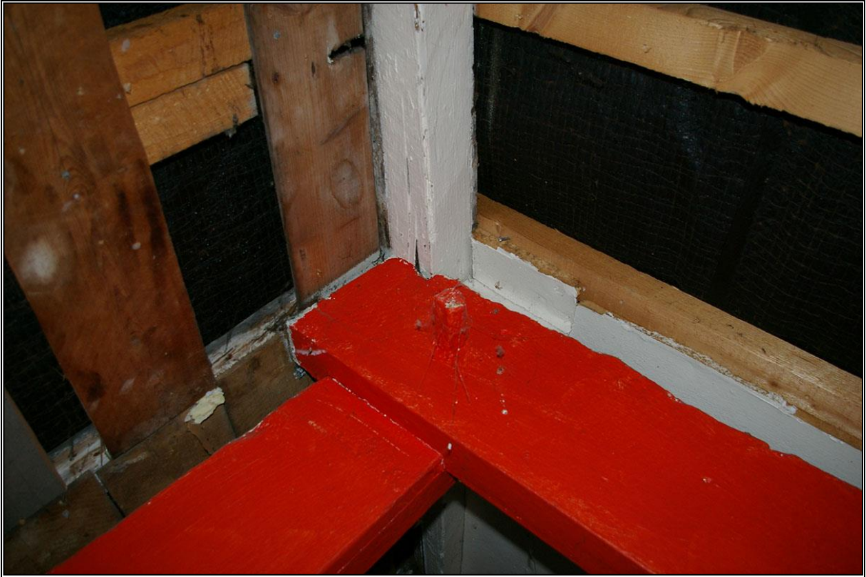
DETAIL OF ONE OF THE PEGGED RIDGES ON THE OLDER 18 TH CENTURY TRUSSES; FROM THE SOUTH.
