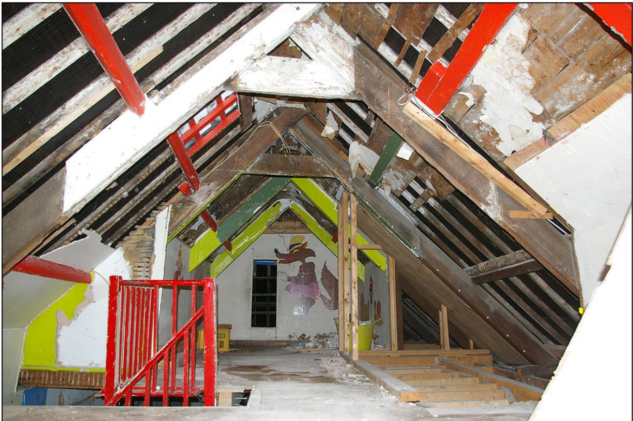
ROOM 10, THE ATTIC, WITH ROOF TRUSSES OF TWO DIFFERENT PHASES; FROM THE NORTH.
