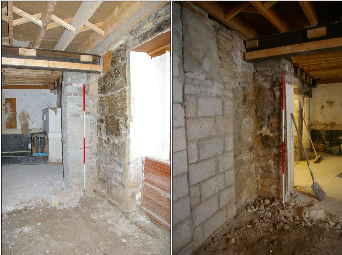
LEFT: THE SOUTH-WEST CORNER OF THE EARLIER BUILDING WITHIN NO.1 NEW STREET, SHOWING THE STUB OF THE ORIGINAL GABLE END WALL; FROM THE NORTH-EAST (2M SCALE).
