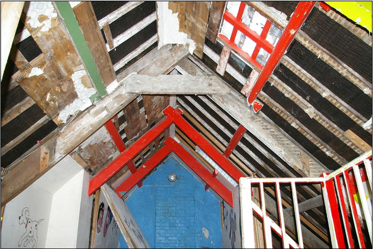
THE THREE HISTORIC PEGGED TRUSSES TO THE NORTH OF NO.1 NEW STREET, IN ROOM 10; FROM THE SOUTH.
