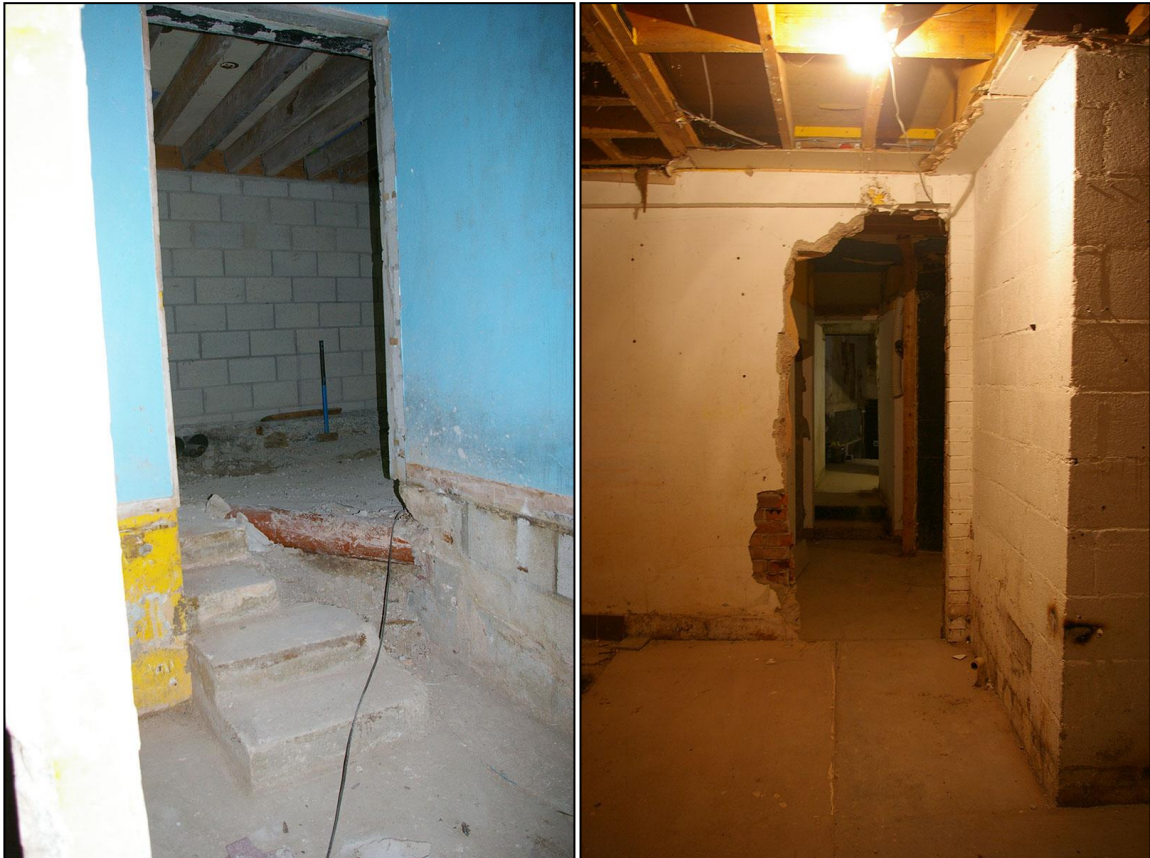
LEFT: ROOM 3B, A MODERN CONCRETE DISABLED TOILET WITHIN THE WEST SIDE OF THE FORMER SYNAGOGUE; FROM THE SOUTH-WEST. RIGHT: FORCED OPENINGS, LOOKING FROM ROOM 4, THROUGH ROOM 3 TO ROOM 2; FROM THE EAST.
