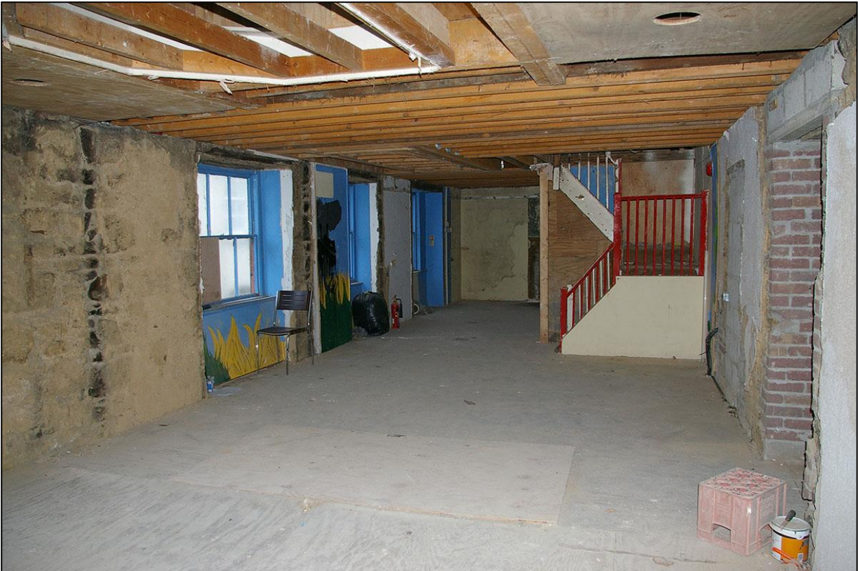
THE FIRST FLOOR OF NO.1 NEW STREET, ROOM 7, TOTALLY STRIPPED OUT, WITH NO CLEAR LAYOUT SURVIVING; FROM THE SOUTH-EAST.
