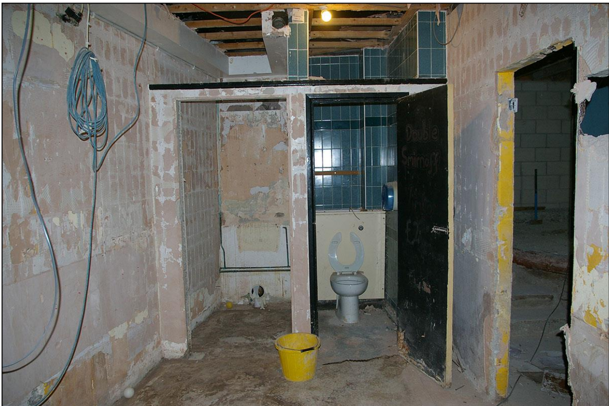
ROOM 3A, A MODERN CONCRETE TOILET BLOCK BUILT IN THE REAR YARD BEHIND NO.1 NEW STREET; FROM THE SOUTH.
