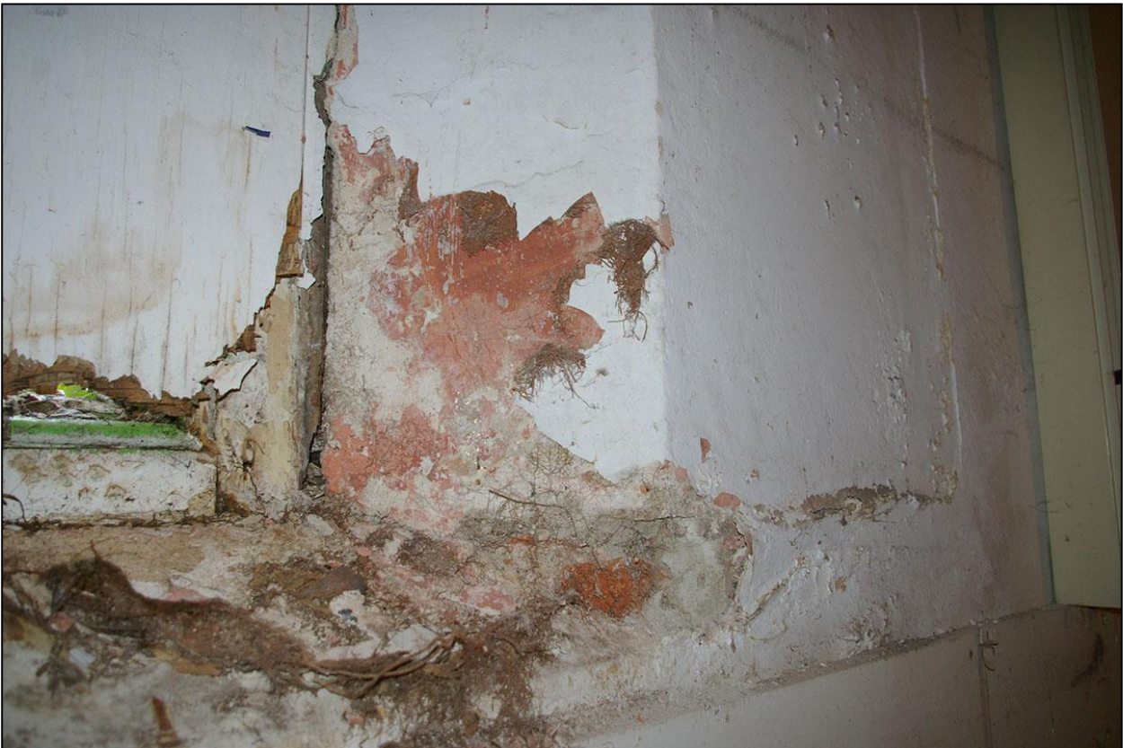
DETAIL OF ONE OF THE WINDOW EMBRASURES, WHERE THE MODERN PLASTER AND PAINT HAVE FALLEN OFF AND EXPOSED AN EARLIER LIME PLASTERED LAYER PAINTED A DARK RED COLOUR.
