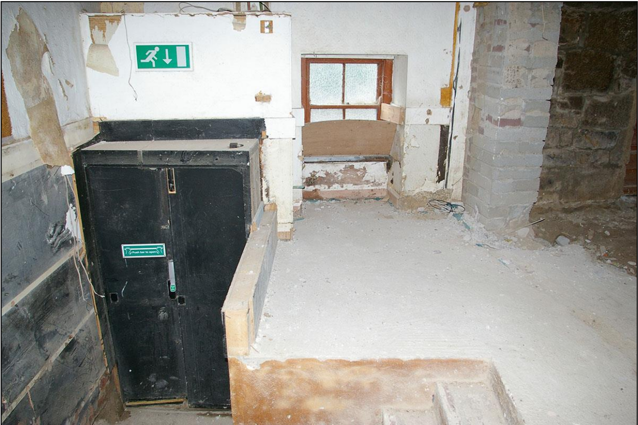
ROOM 1 IN NO.1 NEW STREET, THE BLOCKED CARRIAGE ARCH, WITH INSET DOORWAY ACCESS TO THE DEVELOPMENT SITE AND WINDOW, SHOWING SIGNIFICANT INFILLING BY CONCRETE, TOTALLY ALTERING THE FLOOR LEVELS BY AS MUCH AS 1.5M; FROM THE EAST.
