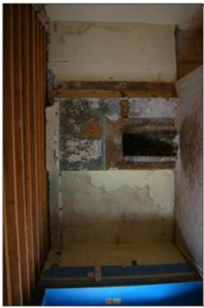
Existing timber and stone floor to be exposed and retained for the new building.
