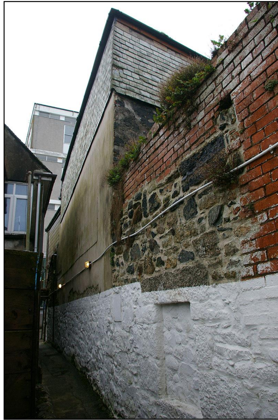
THE SOUTH GABLE END OF THE FORMER SYNAGOGUE, ADJACENT WALL AND BLOCKED WINDOW; FROM THE SOUTH-EAST.
