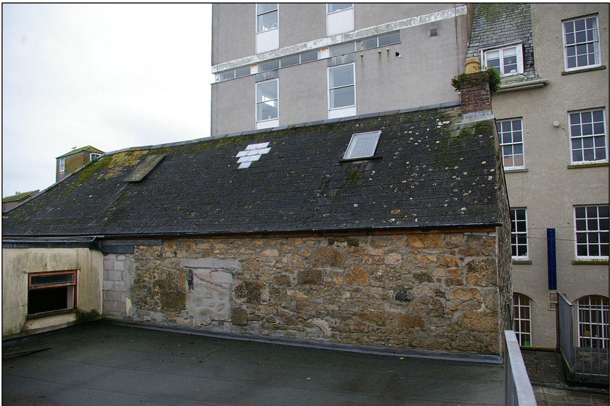
THE EAST WALL OF NO.1 NEW STREET, WITH BLOCKED LOADING DOOR; FROM THE NORTH-EAST.
