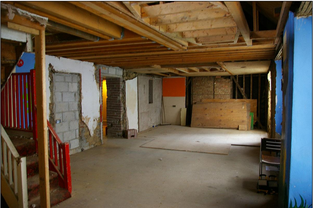
ROOM 7, SHOWING IT HAS BEEN STRIPPED OUT, THE FLOOR AND CEILING REPLACED; FROM THE NORTH-WEST.
