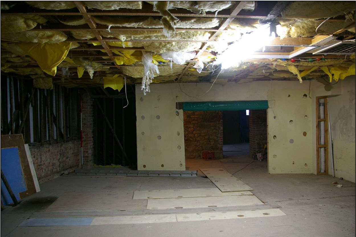
THE WEST WALL OF THE FORMER SYNAGOGUE, ON THE FIRST FLOOR, ROOM 9, SHOWING SIGNIFICANT SECTION TRUNCATED AND REPLACED WITH PLASTERED CONCRETE BLOCK; FROM THE EAST (2M SCALE).
