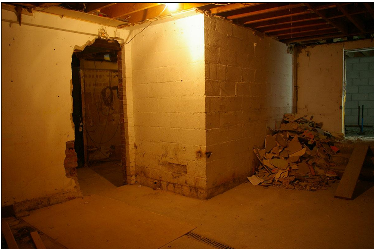
THE CONCRETE INSERTION OF ROOM 3B WITHIN THE FORMER SYNAGOGUE; FROM THE SOUTH-EAST.
