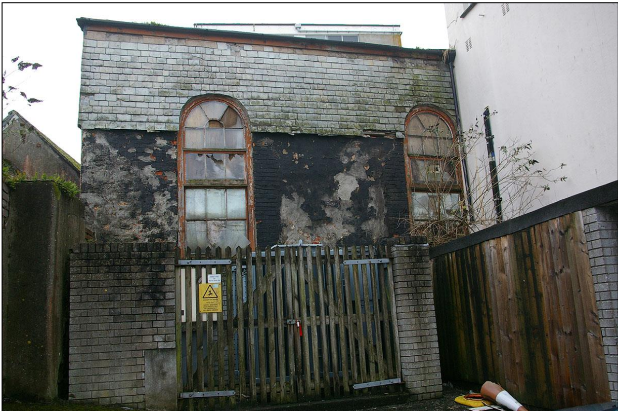
THE EAST ELEVATION OF THE FORMER SYNAGOGUE WITH THE LARGE, ALTERED, ROUND-ARCHED WINDOWS; FROM THE EAST.
