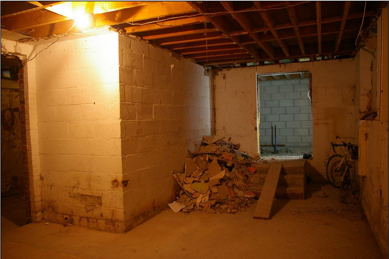
THE FORMER SYNAGOGUE; MODERN STRUCTURES BUILT WITHIN IT, WALLS REMOVED, OPENINGS FORCED AND ALL FITTINGS STRIPPED OUT; FROM THE SOUTH-EAST.
