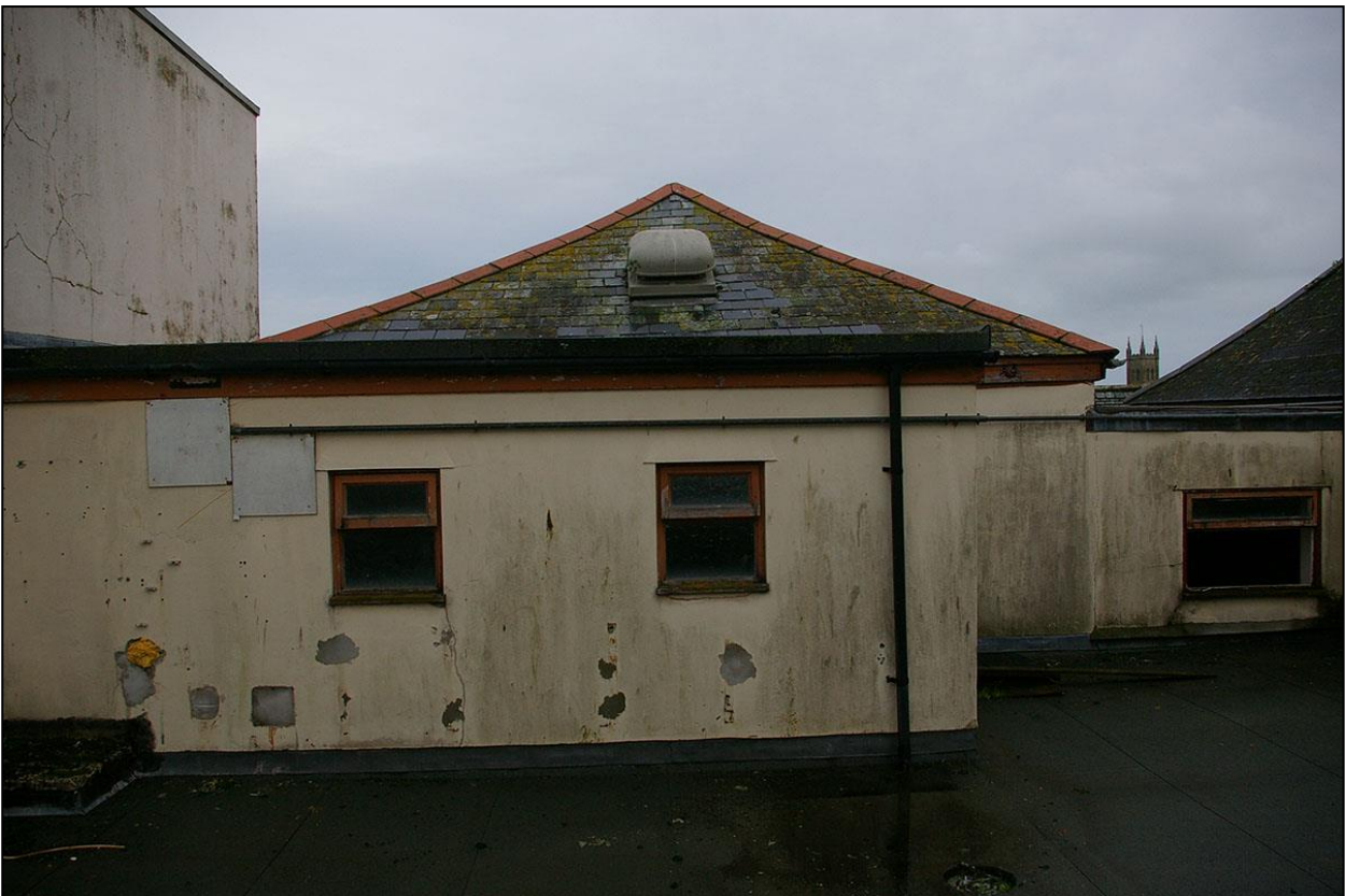
THE HISTORIC COMPOSITE PITCHED ROOF OVER THE SYNAGOGUE, SLATED WITH TERRACOTTA RIDGE TILES; FROM THE NORTH.
