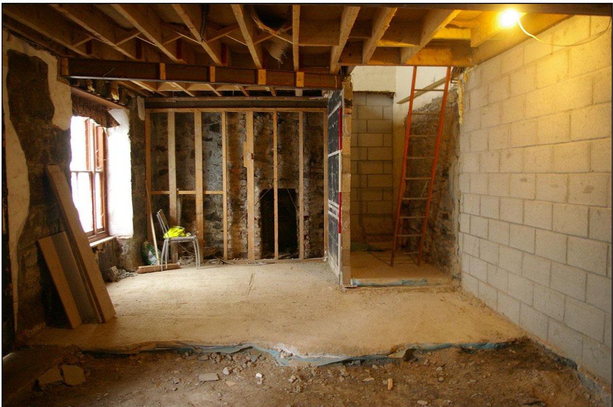
THE NORTH GABLE OF ROOM 1, WITH STONE RUBBLE AND BRICK STACK; FROM THE SOUTH (2M SCALE).
