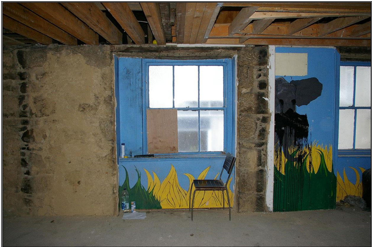
ROOM 7, THE WINDOW TO THE SOUTH, SET WITHIN A PARTIALLY BLOCKED OPENING, THIS PHASING NOT VISIBLE ON THE ASHLAR FRONTAGE; FROM THE EAST.
