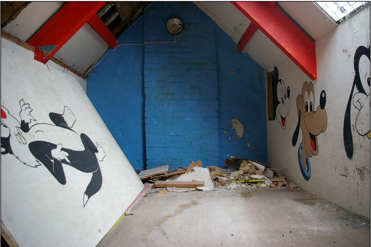
THE UPPER SHALLOW BRICK STACK BUILT ONTO THE NORTH GABLE OF NO.1 NEW STREET; FROM THE SOUTH.
