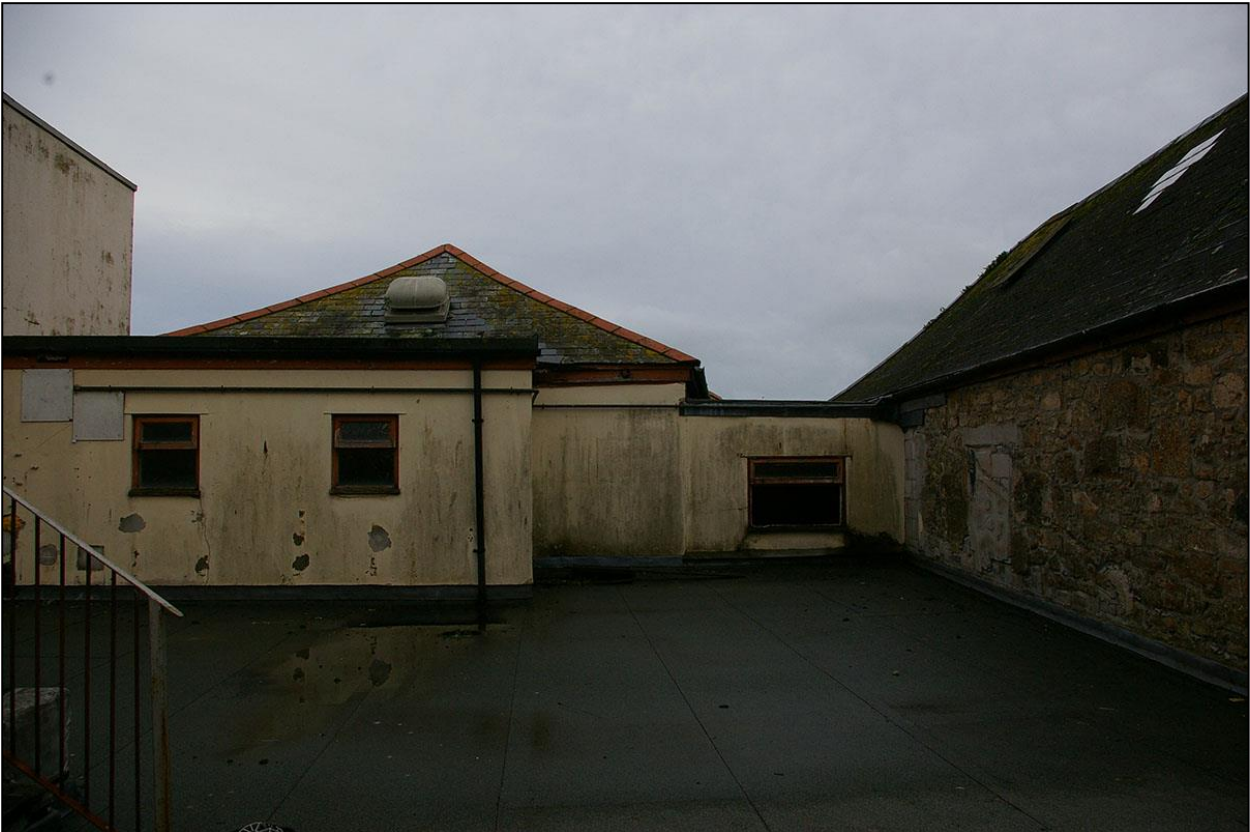
THE FLAT ROOF OVER THE INFILLED COURTYARD BEHIND THE STAR INN, WHICH ABUTS NO.1 NEW STREET AND THE FORMER SYNAGOGUE; FROM THE NORTH.
