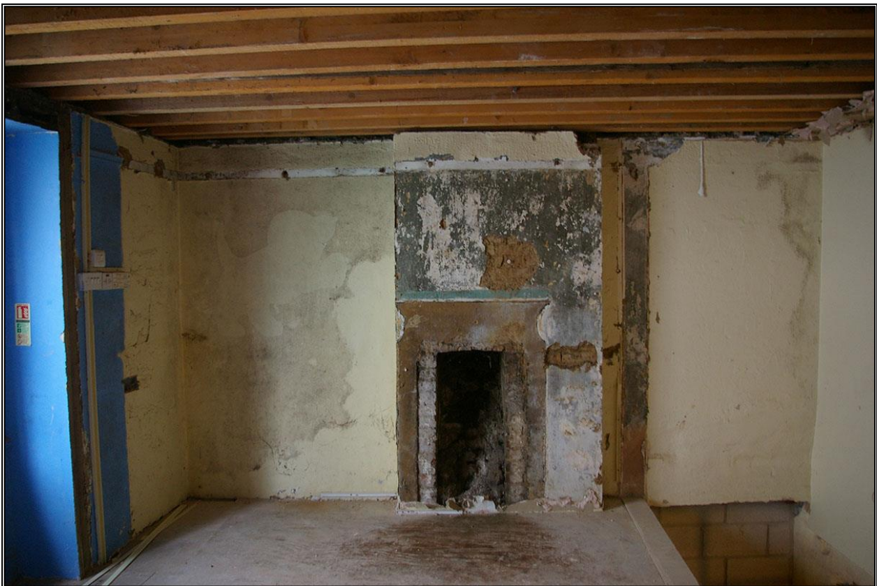
THE NORTH GABLE OF ROOM 7, WITH STONE RUBBLE AND BRICK STACK, PLASTERED HERE, WITH AT LEAST TWO PHASES OF HISTORIC PAINT, GREEN AND BLUE, WITH PARTIALLY BLOCKED FIREPLACE, ALTERED TO FIT A GRATE; FROM THE SOUTH.
