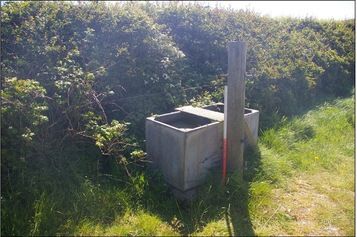
DETAIL OF THE WATER TROUGH BETWEEN FIELDS 1 AND 2; FROM THE NORTH-WEST (1M SCALE).
