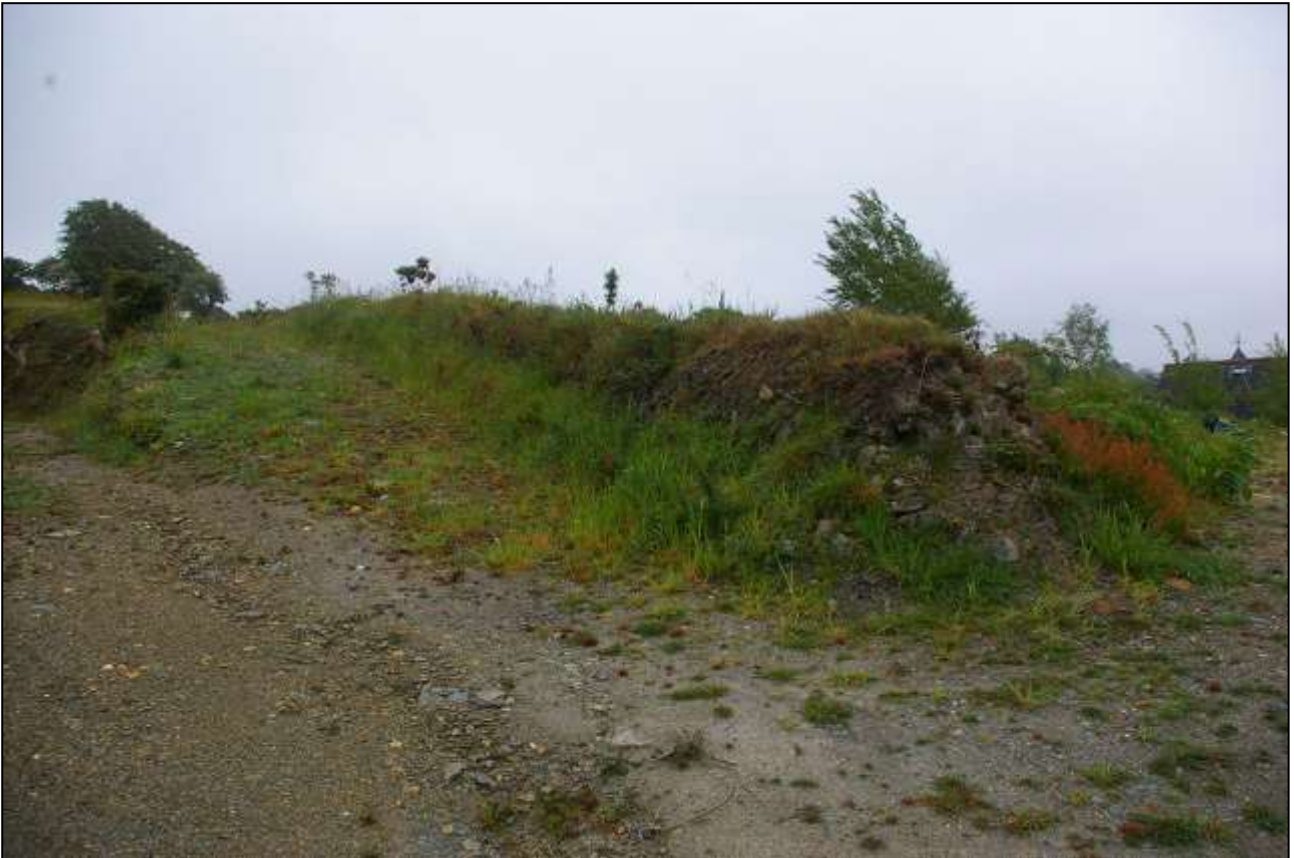
27. VIEW OF THE PART DUMPED EARTH AND QUARRY WASTE; PART HERRINGBONE STONE-FACED SOUTHERN BOUNDARY BANK; FROM THE WEST.
