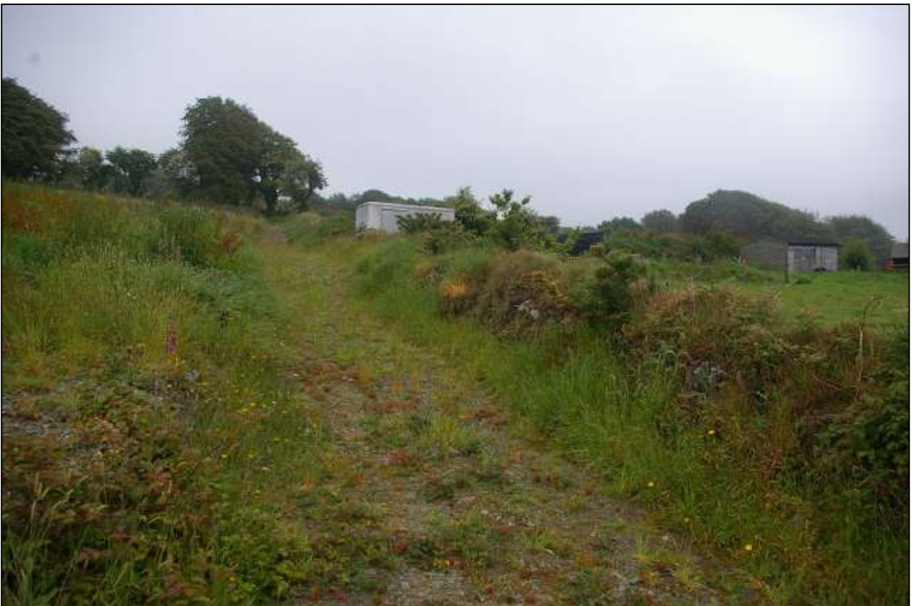
28. VIEW ALONG THE SOUTHERN LOW BANK BOUNDARY, SHOWING THE LOOSE UPLAND GRASS TOPPING AND ABSENCE OF HEDGE; FROM THE WEST, NORTH-WEST.
