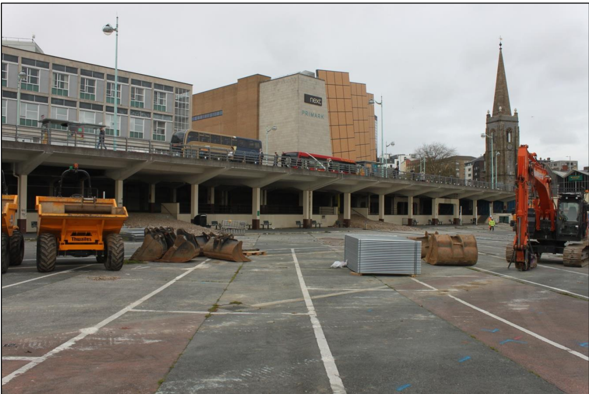
GENERAL SITE SHOT PRIOR TO THE COMMENCEMENT OF GROUNDWORKS; VIEWED FROM THE SOUTH-EAST (NO SCALE).
