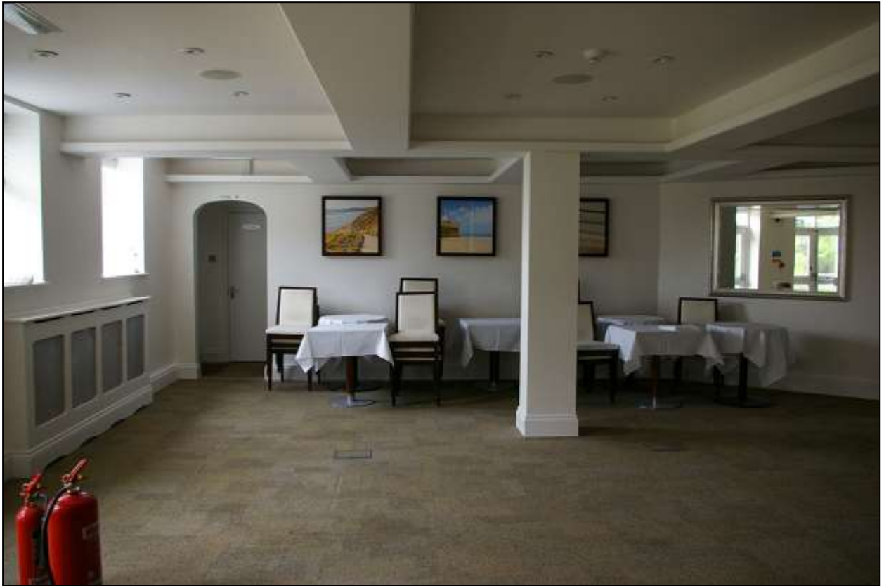
VIEW OF THE NORTHERN PARTITION WALL WHICH FORMS A SET OF TOILETS FOR THE PRIVATE HIRE ROOM THE BASEMENT IS USED AS; FROM THE SOUTH.
