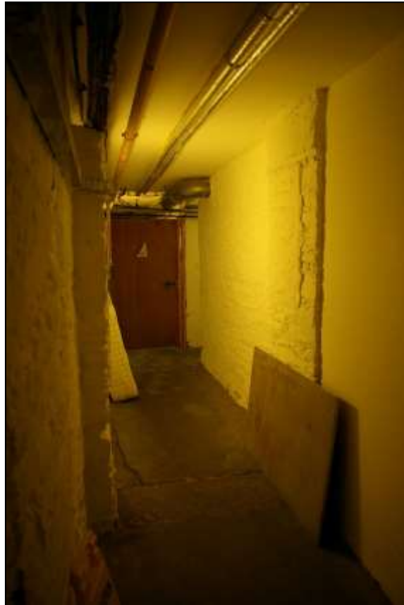
VIEW OF THE BASEMENT CORRIDOR WHERE IT TURNS A CORNER AND OF FORCED STONE WALLS AND MODERN PARTITION WALL WHICH FORM THE CURRENT BASEMENT SERVICE SPACES; FROM THE WEST, NORTH-WEST.
