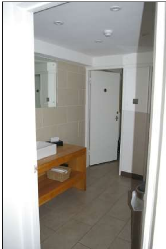
THE TOILETS WITHIN THE PARTITION TO THE NORTH OF THE BASEMENT; FROM THE SOUTH-WEST.
