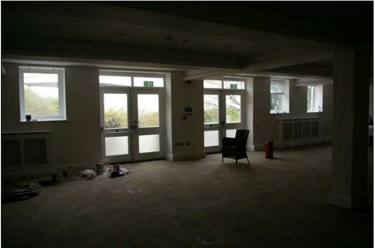
THE FRONT WEST WALL OF THE LOWER BASEMENT, WITH MODERN WINDOWS AND FRENCH DOORS TO THE LOWER TERRACE; FROM THE SOUTH-EAST.
