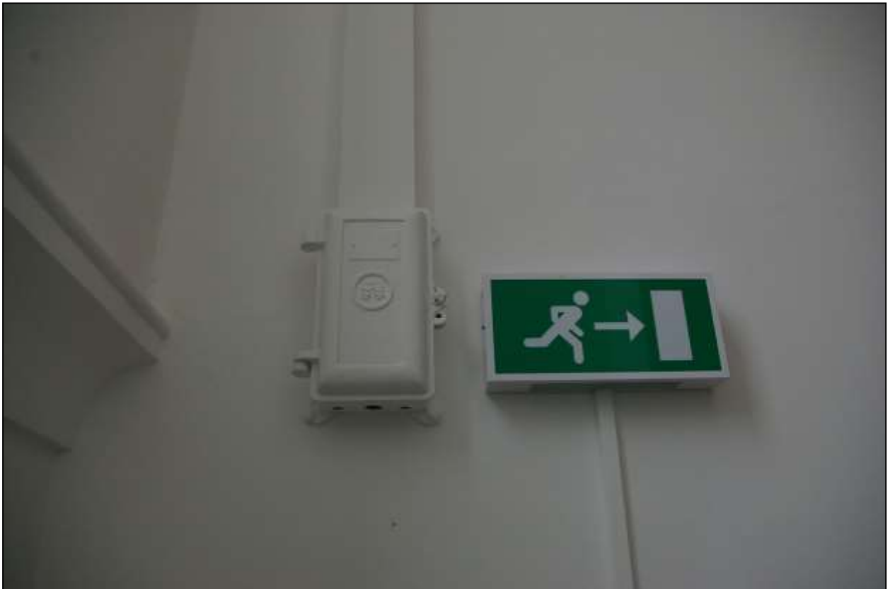
HISTORIC ELECTRIC UNIT ON THE STAIRS TO THE BASEMENT; FROM THE SOUTH.
