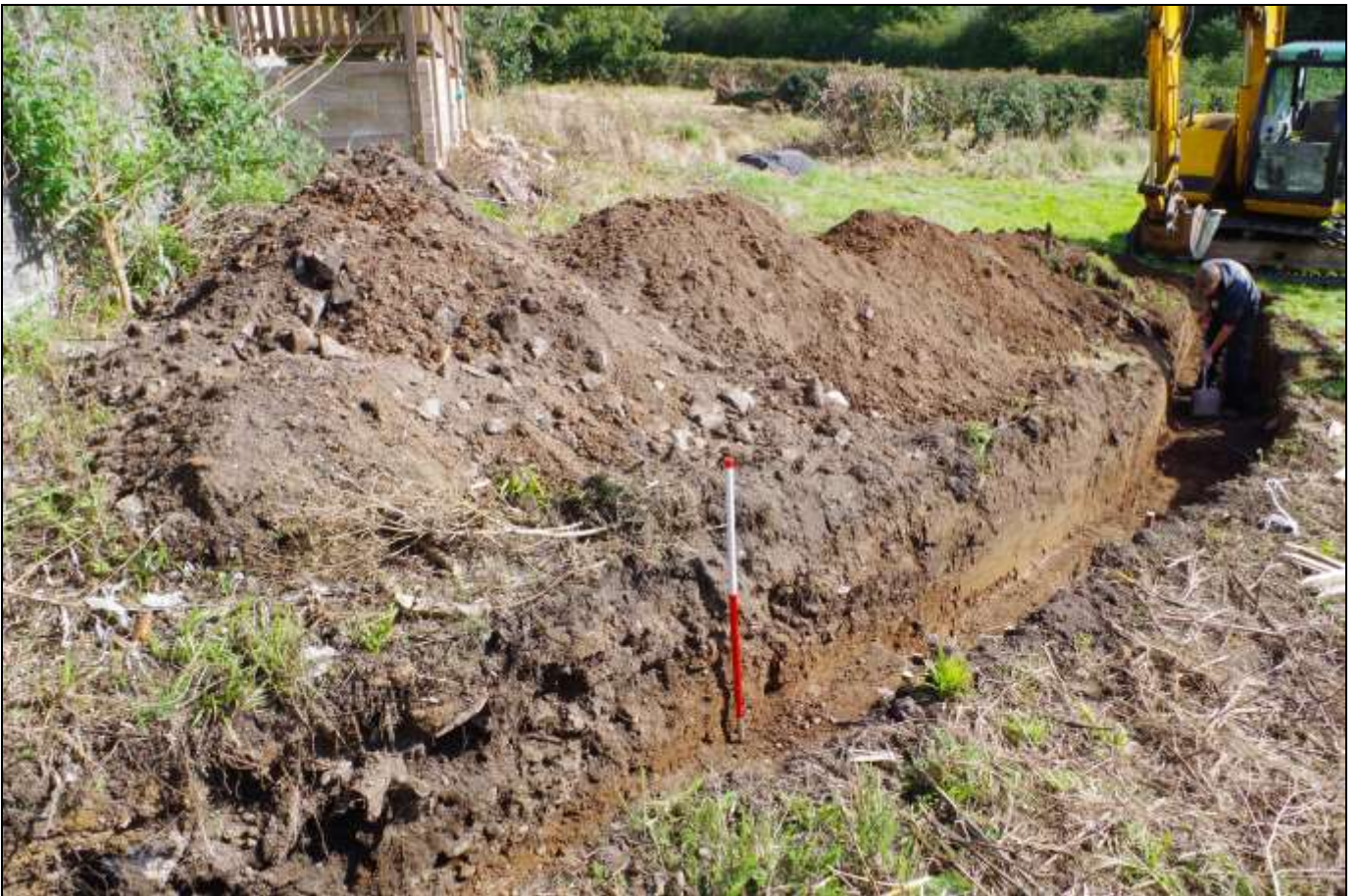
FIGURE 4: FOOTING TRENCH DURING EXCAVATION, THE SCALE LOCATED IN THE LOCATION OF THE BURIED BANK (106); VIEWED FROM THE NORTH-EAST (1M SCALE).
