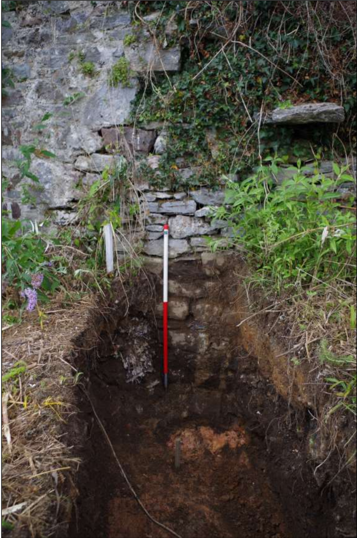
FIGURE 2: EXPOSED STONE WALL FOOTING, NOTE THE PROJECTING STONE IN THE BUILD ABOVE, POTENTIALLY FOR A SLUICE(?), VIEWED FROM THE EAST (1M SCALE).
