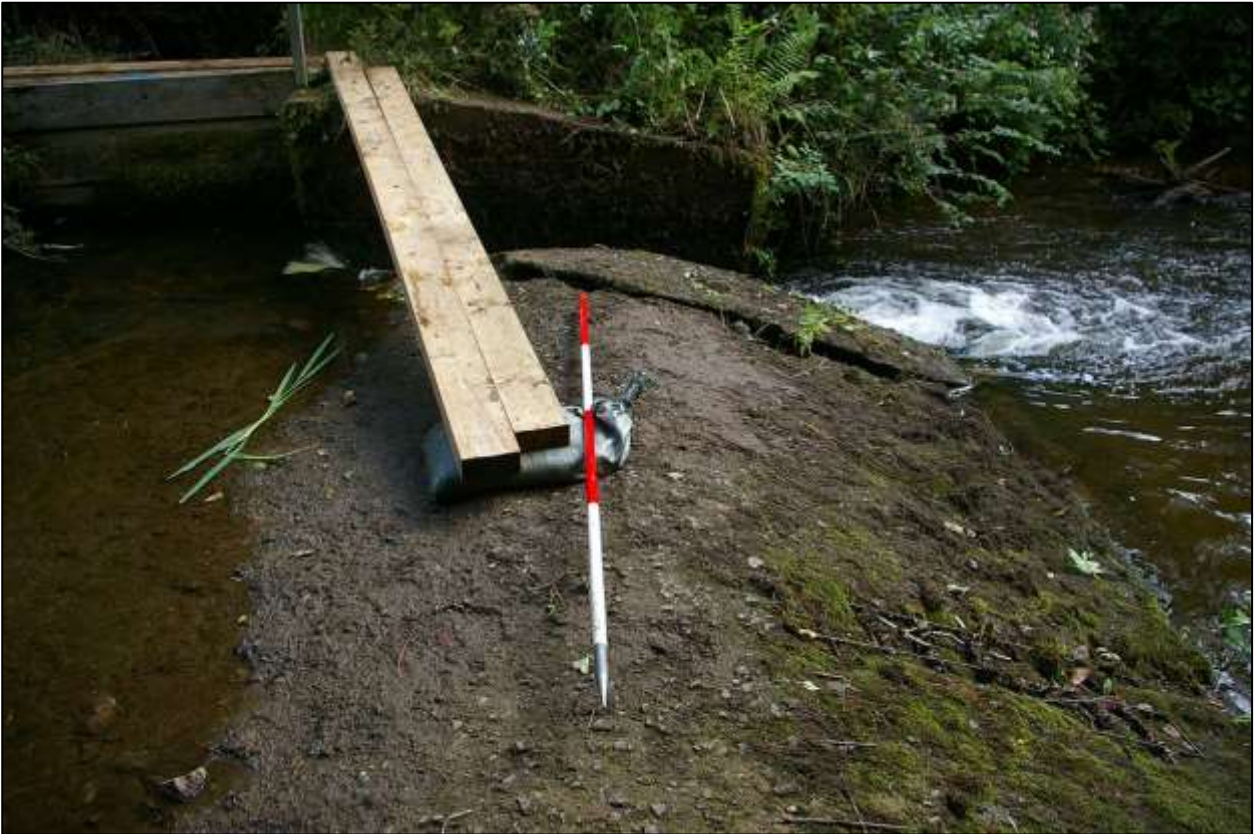
34. THE CONCRETE CAP OF THE WEIR, WITH WATER DRAINED OFF, SHOWING A RELATIVELY MODERN TOP-COAT, HELD IN PLACE BY STEEL SQUARE MESH; WITH 2M SCALE; FROM THE EAST-SOUTH-EAST.
