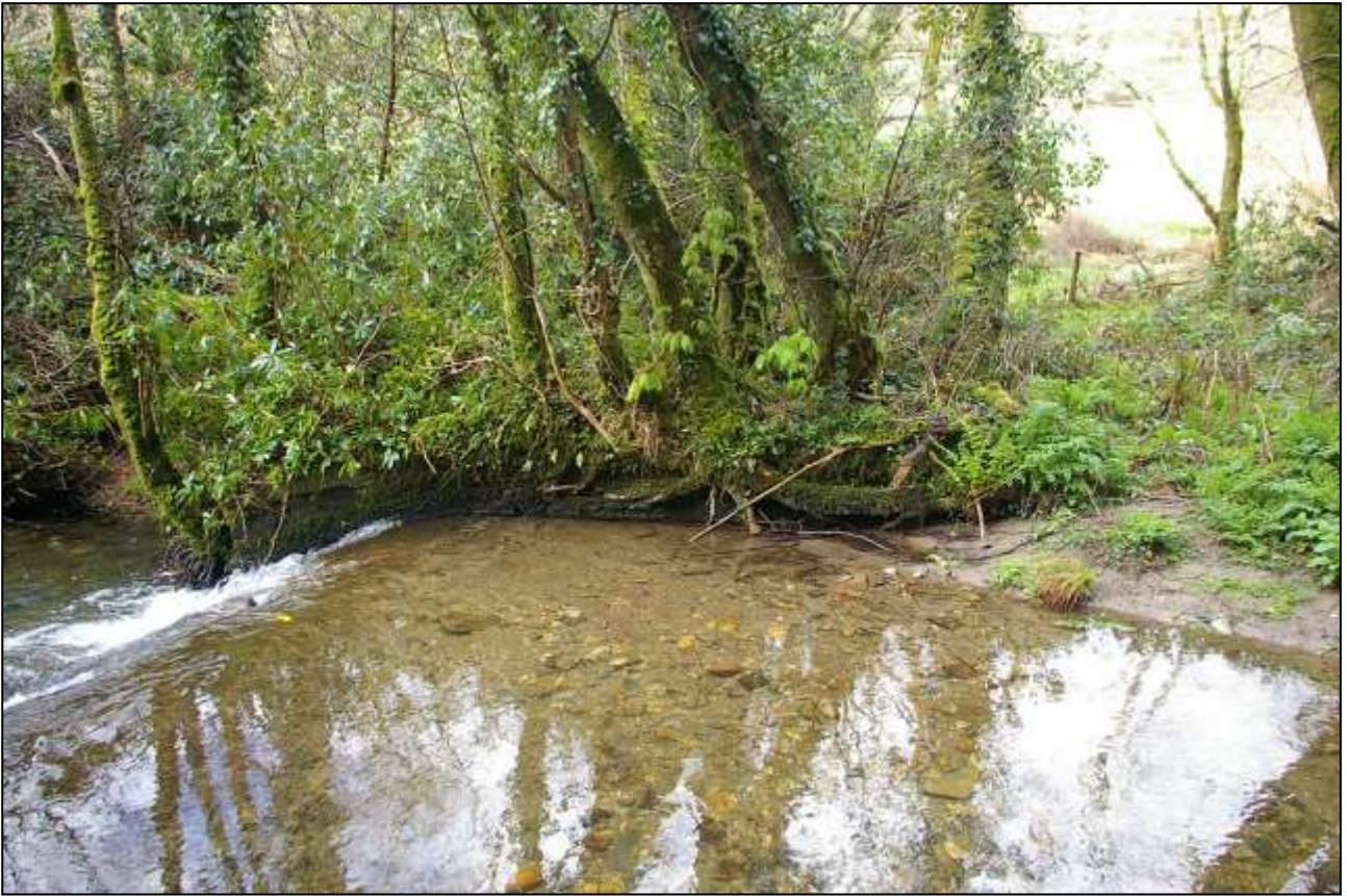
7. THE WESTERN ABUTMENT OF THE WEIR, SHOWING DARK COLOURED, COURSED STONEWORK, TOPPED BY A CEMENT CAP; FROM THE EAST, NORTH-EAST.
