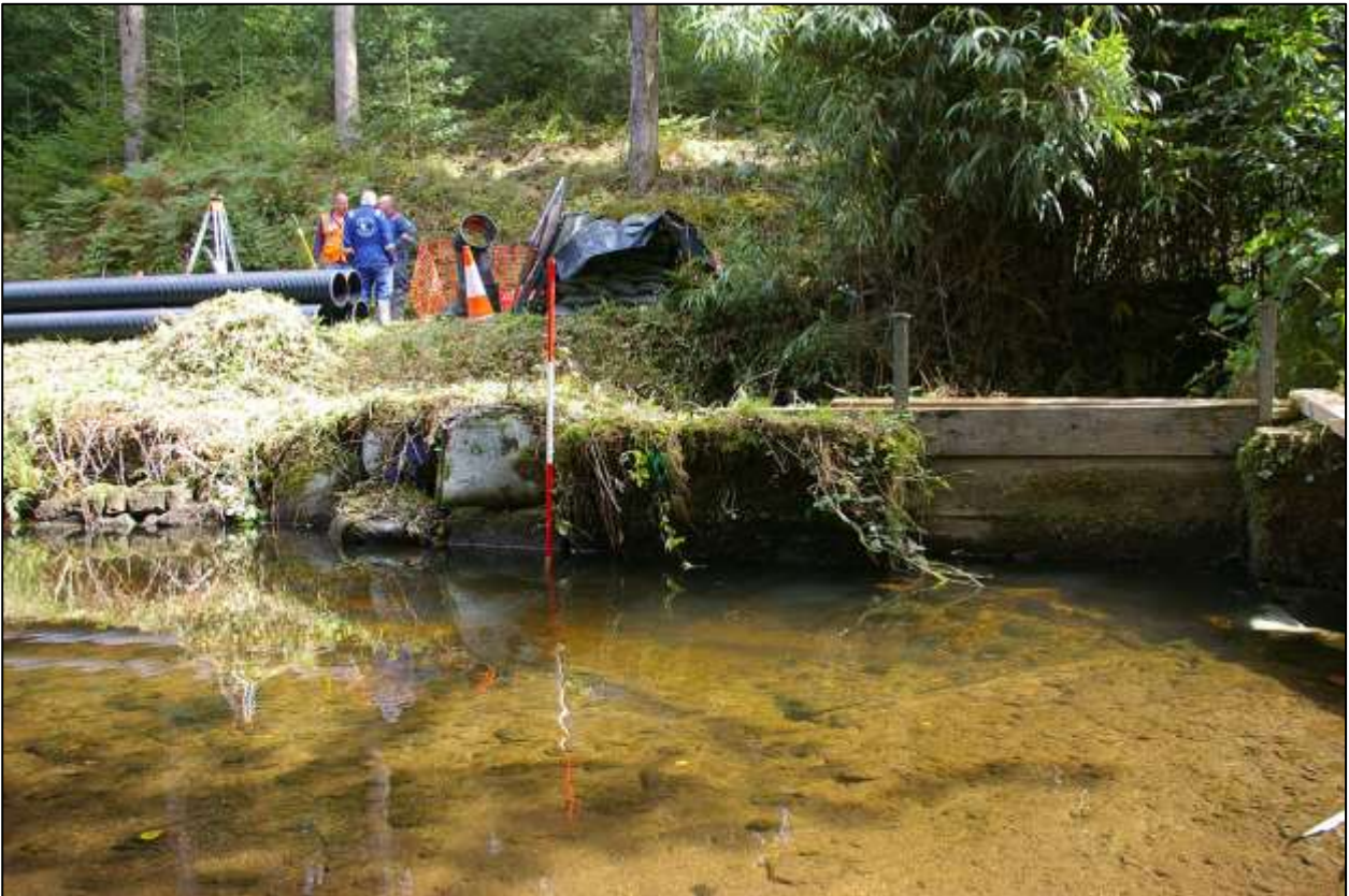
30. THE FLANK WALL OF THE LEAT AND SLUICE GATE, SHOWING ITS REPAIR WITH DUMPY BAGS FULL OF RUBBLE AND ROCKS, WITH SOME CEMENT PATCHING; WITH 2M SCALE; FROM THE SOUTH-WEST.
