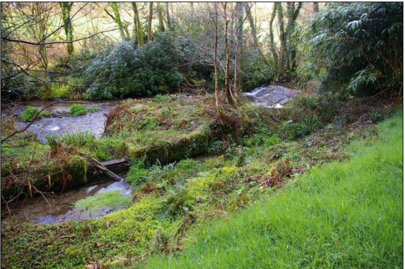
14. WIDE ANGLED VIEW OF THE WEIR, RIVER, LEAT AND OVERFLOW GATE; FROM THE EAST, SOUTH-EAST.
