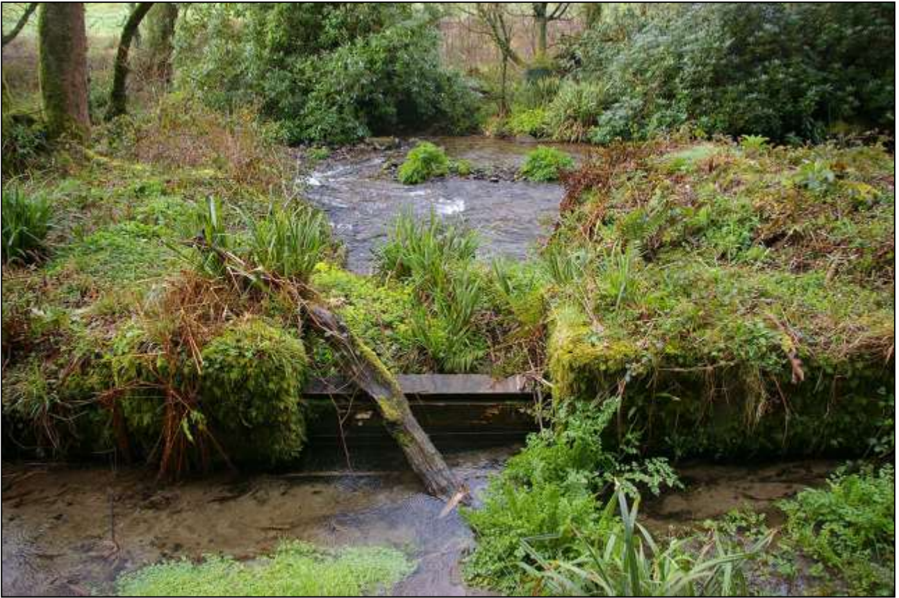
15. THE SILTED UP OVERFLOW GATE TO THE LEAT; FROM THE EAST.
