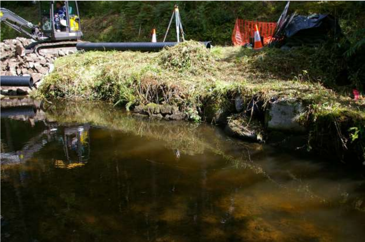
40. LONG VIEW OF THE RIVER BANK, RUNNING NORTH AWAY FROM THE WEIR, UPSTREAM, SHOWING A SMALL SECTION OF MORTARED ROUGH BLOCKS, WHICH ARE COMING FREE FROM THE BANK, SHOWING THE SCOURING PROBLEM ON THE EASTERN SIDE OF THE RIVER HERE; FROM THE SOUTH-SOUTH-WEST.
