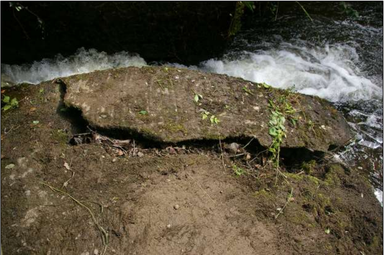
38. THE LARGE CRACK IN THE CONCRETE, TO THE EAST END OF THE WEIR; FROM THE WEST.
