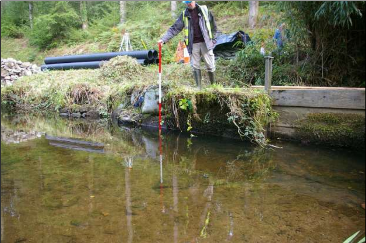
32. THE SHORT SECTION OF GOOD FLANK WALL TO THE SLUICE, COVERED IN CEMENT RENDER, WITH 2M SCALE; FROM THE SOUTH-WEST.
