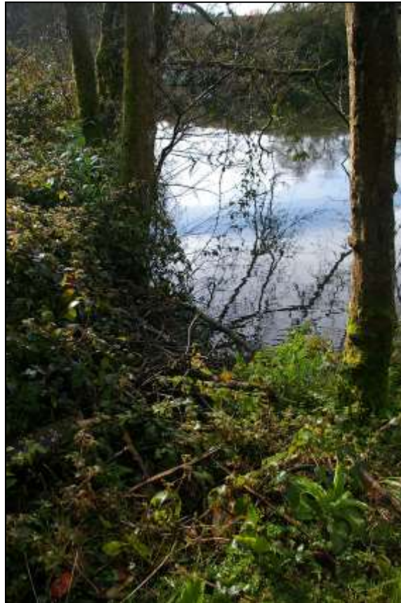
20. THE CULVERT WHICH CARRIES THE LEAT WATER INTO THE LAKE, IN ITS NORTH-EAST CORNER, INFILLED WITH FALLEN TWIGS AND BRANCHES; FROM THE NORTH-WEST.
