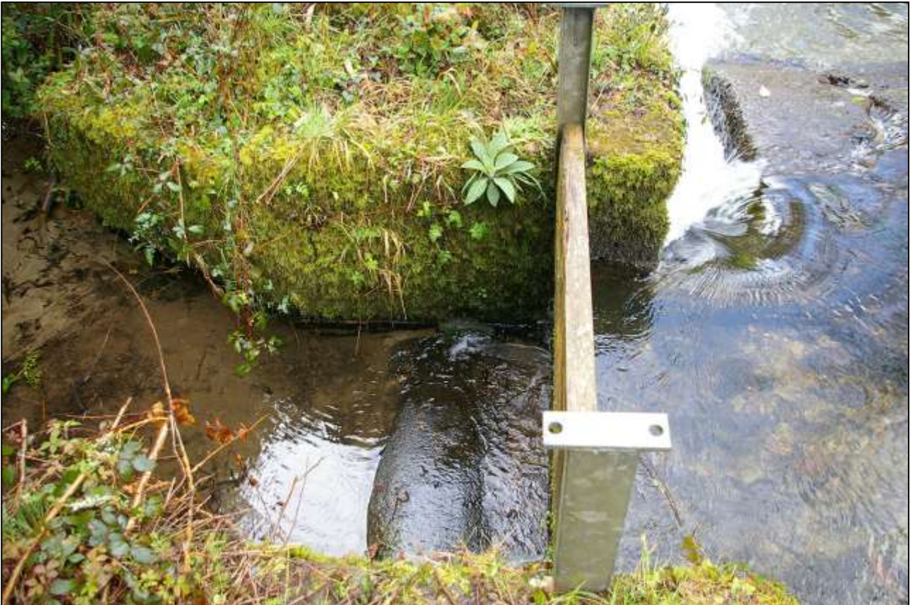
9. THE SLUICE GATE TO THE WORKING LEAT, WITH GALVANISED I-PROFILE GIRDERS AND MODERN BOARDS, FIXED WITH CEMENT TO OLDER STONE AND CONCRETE CAPPED ABUTMENT WALLS; FROM THE NORTH.
