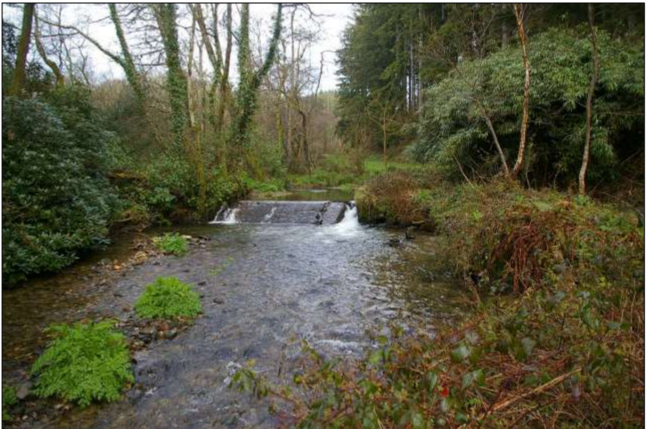
27. VIEW OF THE WEIR AND ANGLED EASTERN ABUTMENTS, WITH OVERFLOW GATE; FROM THE SOUTH.
