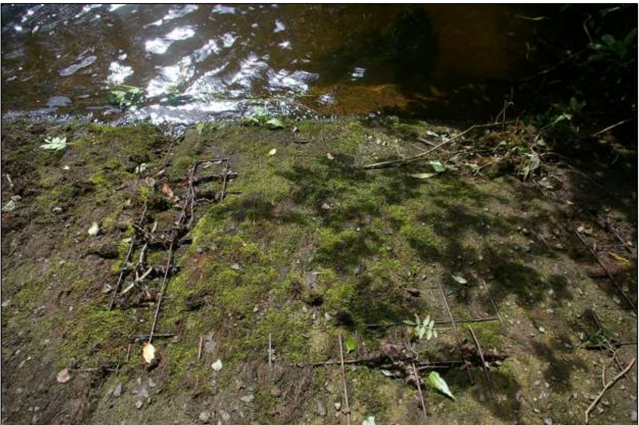
37. DETAIL OF THE STEEL MESH WHICH IS HOLDING THE UPPER CONCRETE CRUST OVER THE DAM, CLEARLY A FAIRLY RECENT REPAIR TO THE STRUCTURE; FROM THE NORTH-NORTH-WEST.
