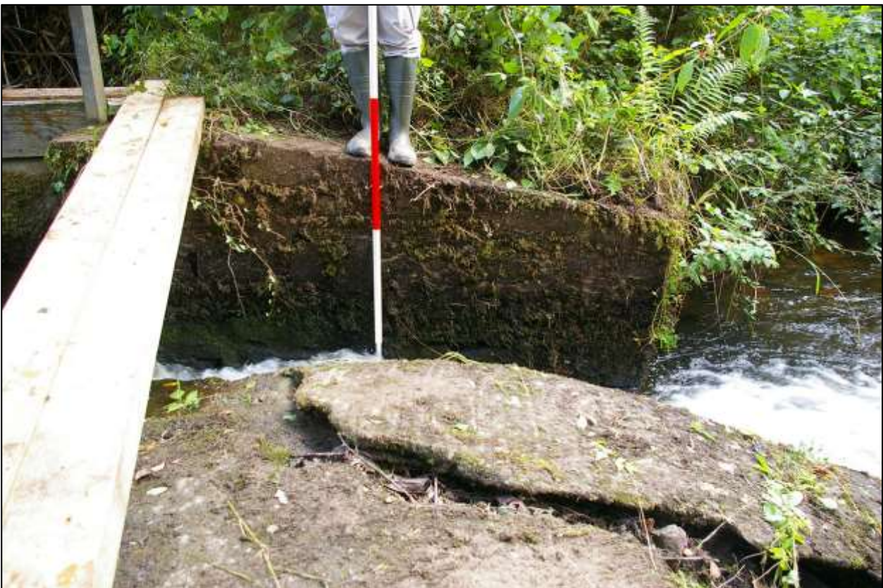
33. THE LOWER ANGLED SECTION OF FLANK WALL, WHICH BRACES THE WEIR, OF DRESSED SLATESTONE BLOCKS AND CEMENT RENDER CAPPING AND SIDES; WITH 2M SCALE; FROM THE WEST-SOUTH-WEST.
