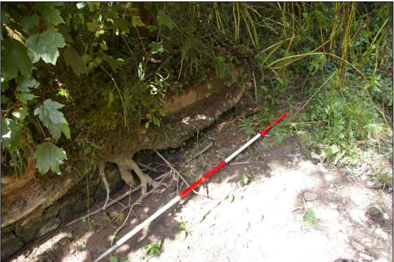
39. DETAIL SHOWING THE MASSIVE ROOT OF A TREE WHICH HAS GROWN INTO THE WEST FLANK WALL OF THE WEIR STRUCTURE, WITH 2M SCALE; FROM THE EAST-SOUTH-EAST.
