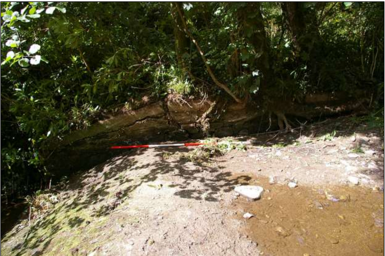
35. THE WEST FLANK WALL TO THE WEIR, SHOWING HEAVY BLOCK CONSTRUCTION, CAPPED WITH CONCRETE, WITH THICK POORLY EXECUTED CEMENT REPOINTING; WITH 2M SCALE; FROM THE EAST.
