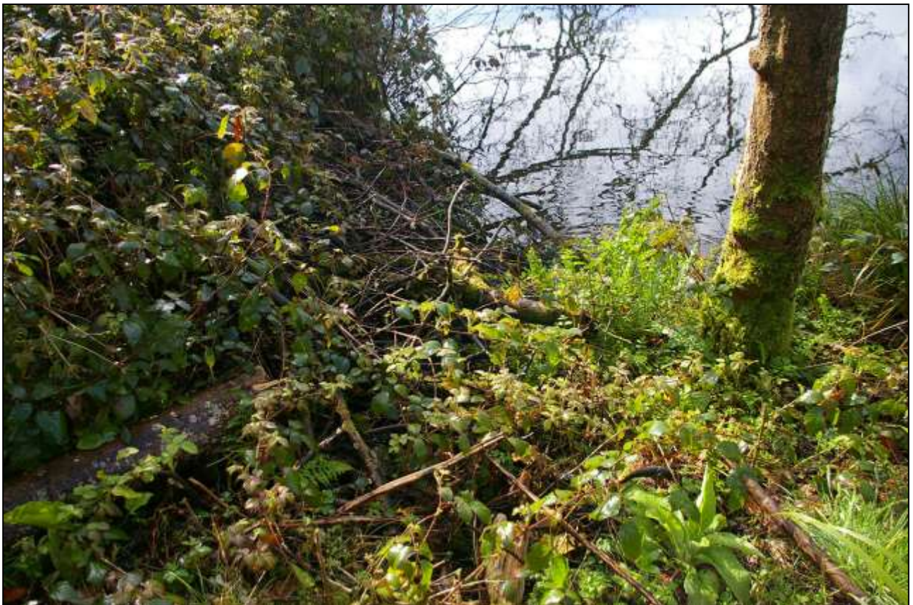
21. CLOSER VIEW OF THE PART OBSCURED CULVERT WHICH FEEDS THE LAKE; FROM THE NORTH, NORTH-WEST.
