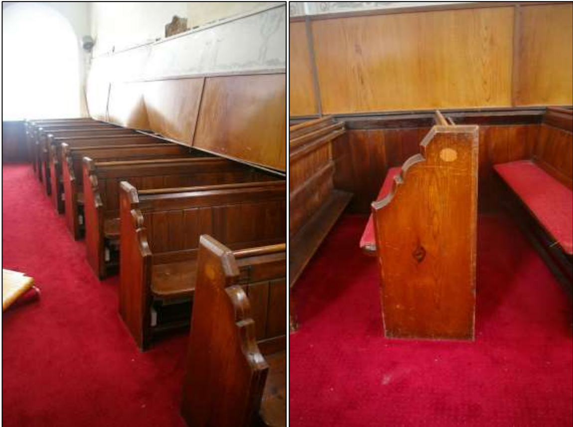
42. LEFT: VIEW OF THE PEWS TO THE WEST, AN EXAMPLE OF THEIR STYLE AND FORM; FROM THE NORTH.
