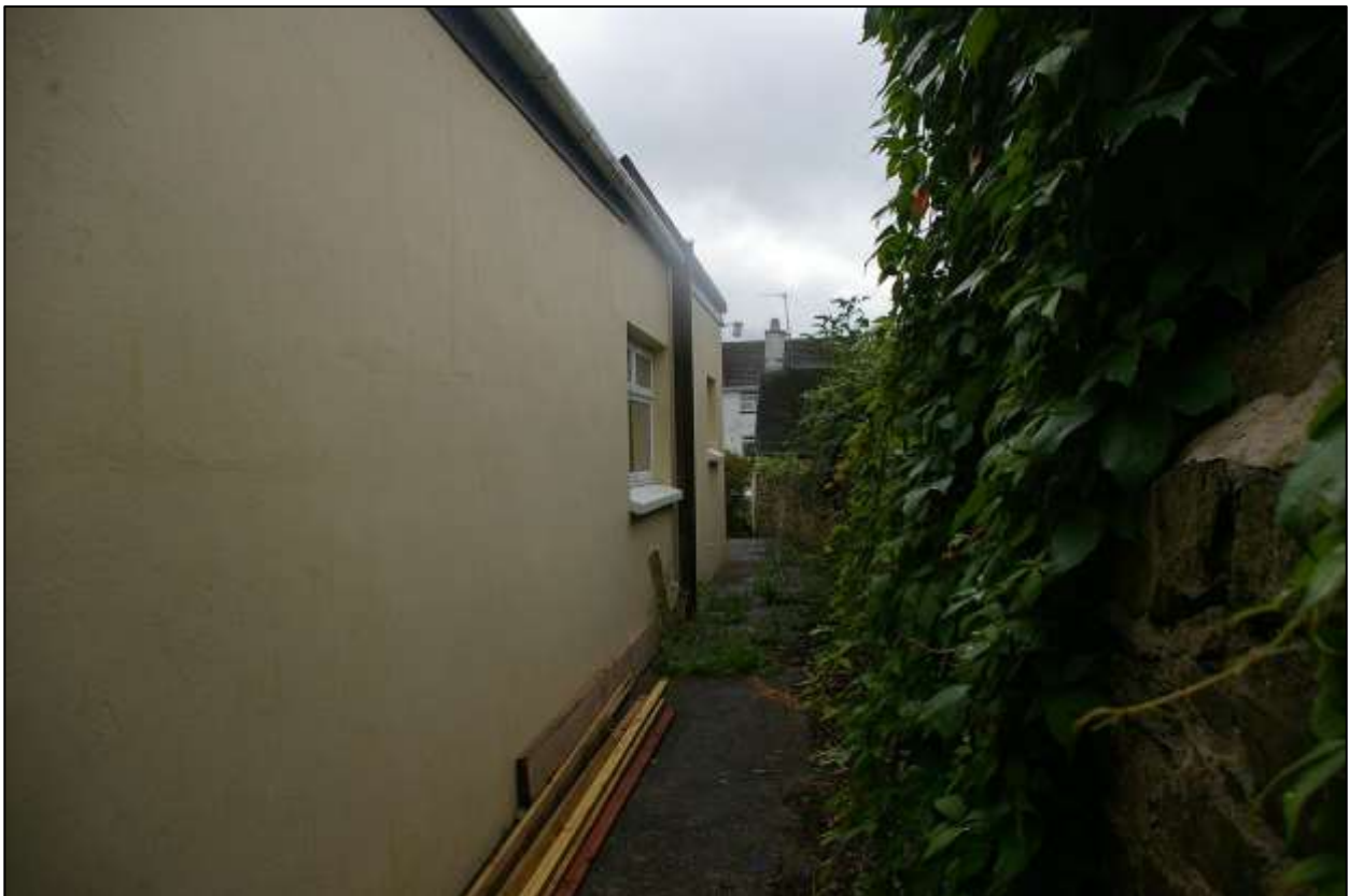
17. THE WEST SINGLE STOREY ELEVATION OF THE COMMUNITY HALL BUILDING; FROM THE NORTH-WEST.
