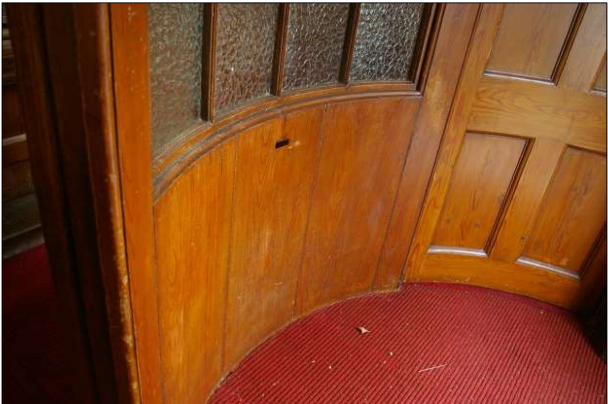
25. THE BEADED PLANK STRUCTURE OF THE WEATHER PORCH AND SLOT FOR THE COLLECTION BOX BUILT INTO IT; FROM THE WEST.
