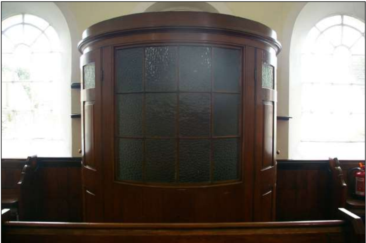
27. THE 12 PANE PANEL IN THE NORTH SIDE OF THE WEATHER PORCH, LIGHTING IT FROM THE AUDITORIUM; FROM THE NORTH.
