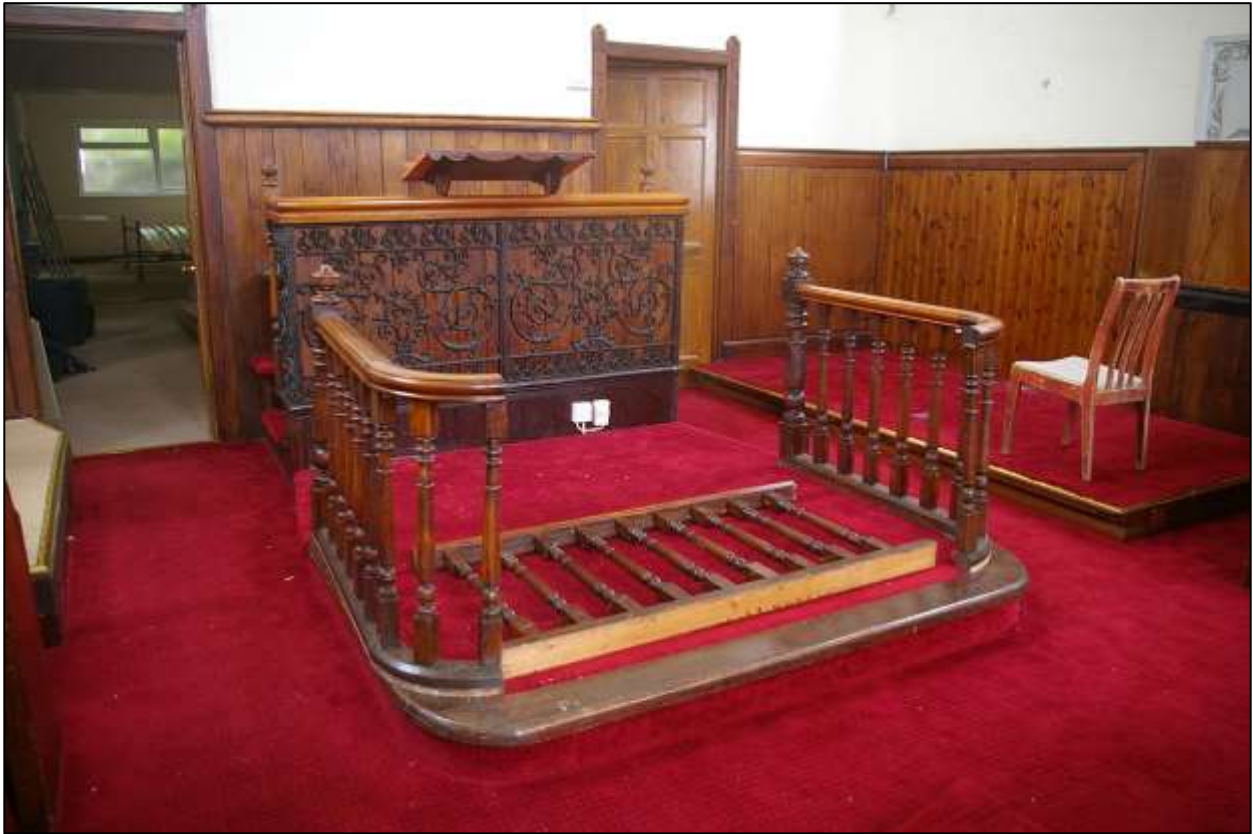
45. THE PULPIT AND RAISED DAIS WITH COLLAPSED COMMUNION RAIL; FROM THE SOUTH-WEST.
