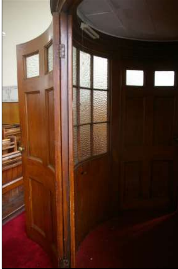
24. THE SEMI-CIRCULAR WEATHER PORCH STRUCTURE, A FINE REGENCY DETAIL; FROM THE WEST, SOUTH-WEST.
