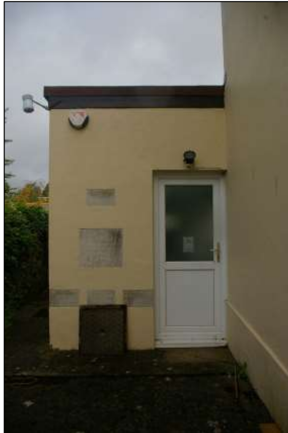
10. D8 – THE REAR ENTRANCE TO THE 1949 COMMUNITY HALL, NOW A MODERN WHITE PVC DOUBLE-GLAZED DOOR. ON THE SOUTH-WEST CORNER ARE A SERIES OF COMMEMORATIVE LIMESTONE PLAQUES TO MEMBERS OF THE CONGREGATION; FROM THE SOUTH.
