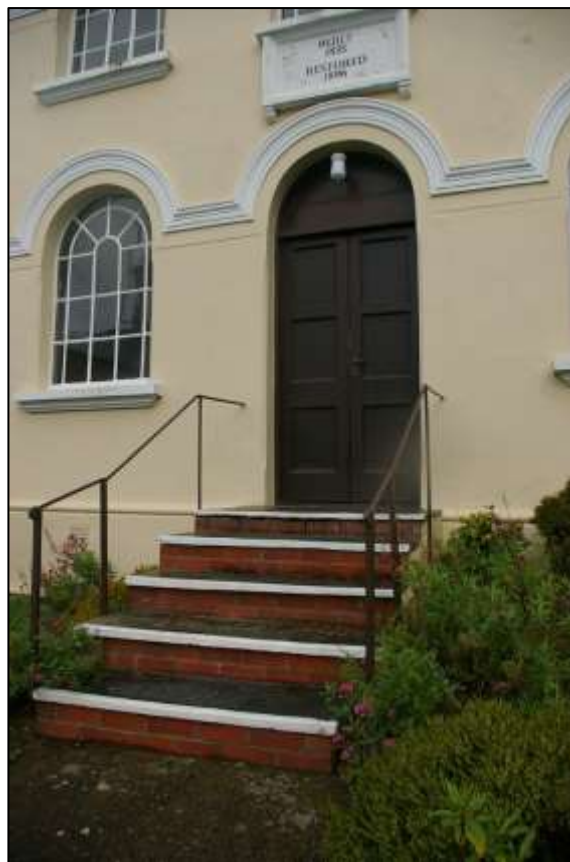
6. THE STEPS UP TO THE FRONT DOOR (D1), THE ORIGINAL SLATES LAID OVER A REPLACEMENT BRICK STRUCTURE; FROM THE SOUTH-EAST.
