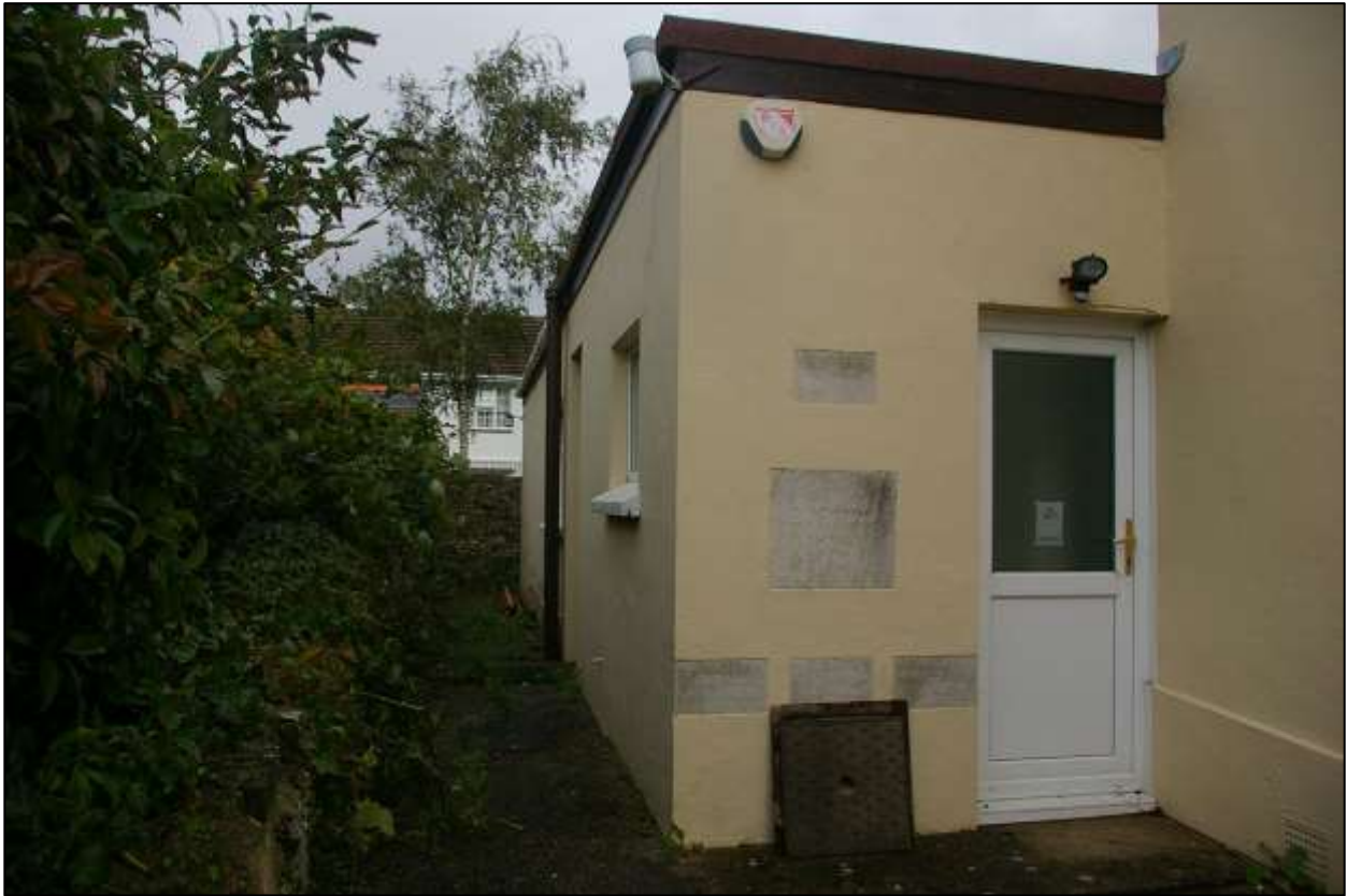
16. THE SOUTH-WEST CORNER AND WEST ELEVATION OF THE LARGE SINGLE STOREY 1949 BUILT COMMUNITY HALL; FROM THE SOUTH, SOUTH-WEST.
