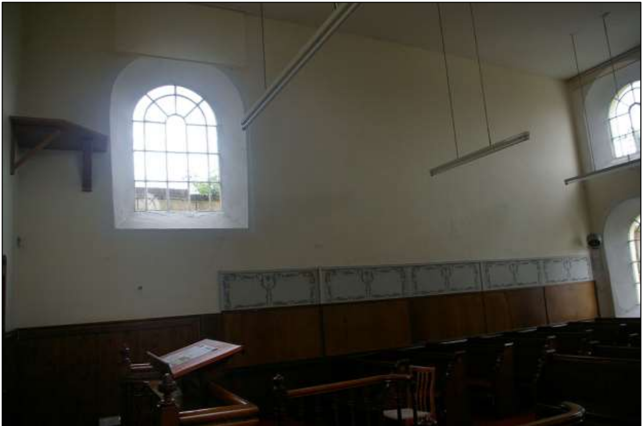
39. THE EAST WALL OF THE CHAPEL, INTERIOR FACE, SHOWING THE WINDOW TO THE NORTH, WHICH APPEARS TO BE THE ONLY ONE ON THIS SIDE; FROM THE NORTH-WEST.
