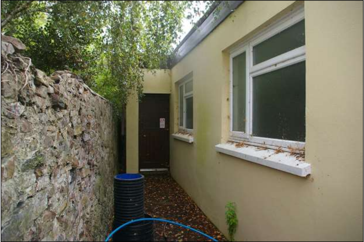
18. THE NORTH ELEVATION OF THE COMMUNITY HALL BUILDING AND REAR FIRE ESCAPE DOOR (D13); FROM THE WEST.
