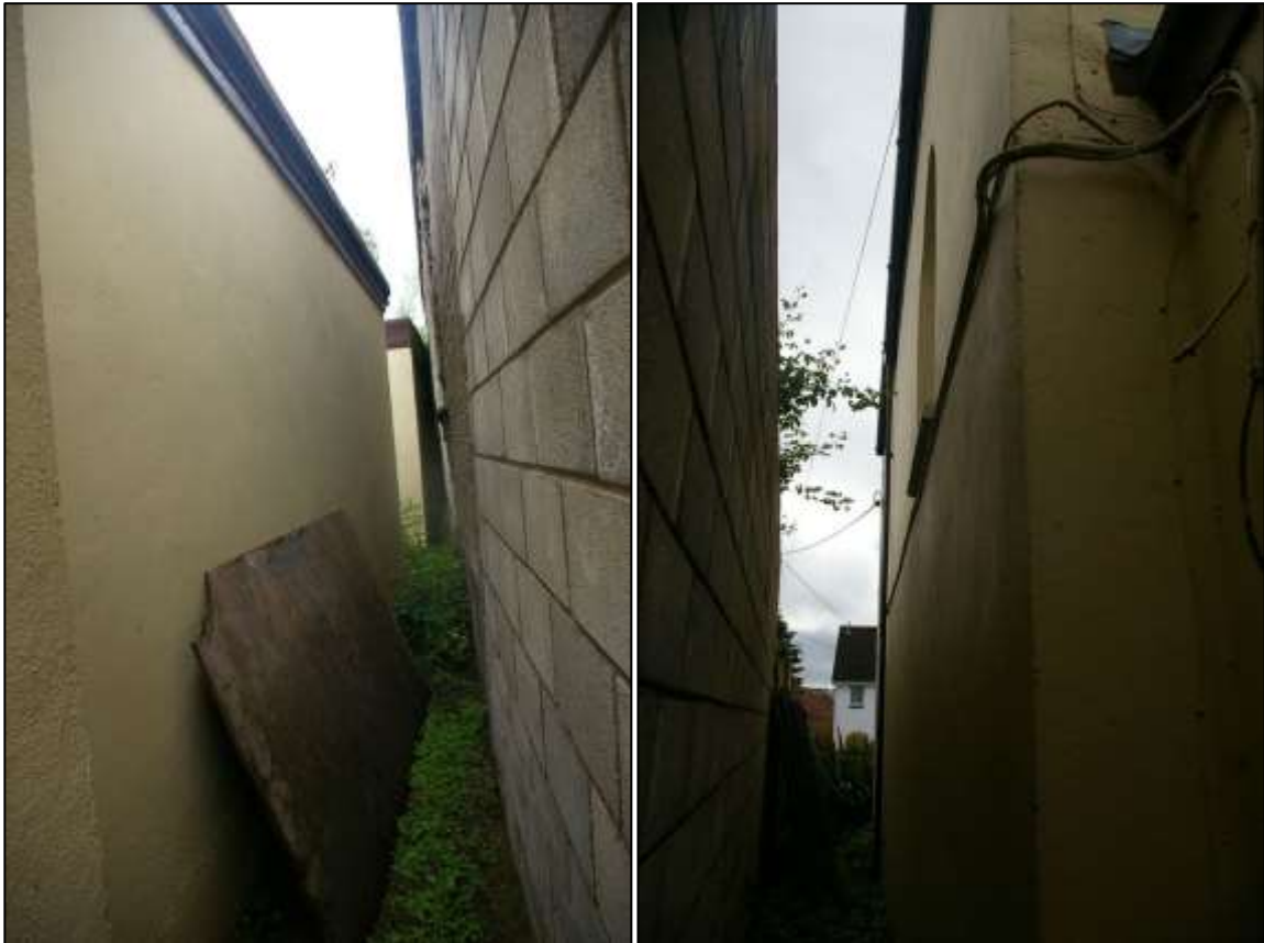
20. LEFT: THE TWO SECTIONS OF THE EAST WALL OF THE COMMUNITY HALL BUILDING; FROM THE SOUTH, SOUTH-EAST. 21. RIGHT: THE EAST WALL OF THE CHAPEL BUILDING, SHOWING THE SINGLE WINDOW OPENING; FROM THE NORTH, NORTH-EAST.
