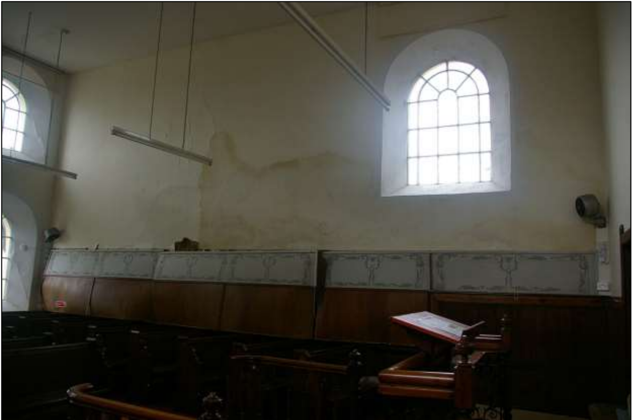
34. VIEW OF THE WEST WALL OF THE CHAPEL, THE INTERIOR FACE, SHOWING THE SURVIVING WINDOW AND MODERN PANELS ABOVE THE PINE PLANK PANELLING, AS WELL AS THE DAMP DAMAGE; FROM THE NORTH-EAST.
