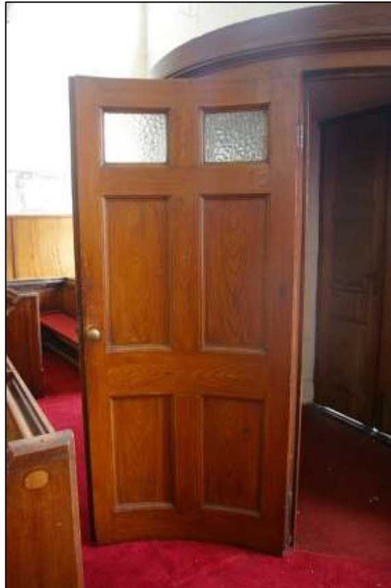
26. D2, SHOWING THE FLAT PANELS ON THE PORCH SIDE OF THE DOORS; FROM THE WEST, NORTH-WEST.
